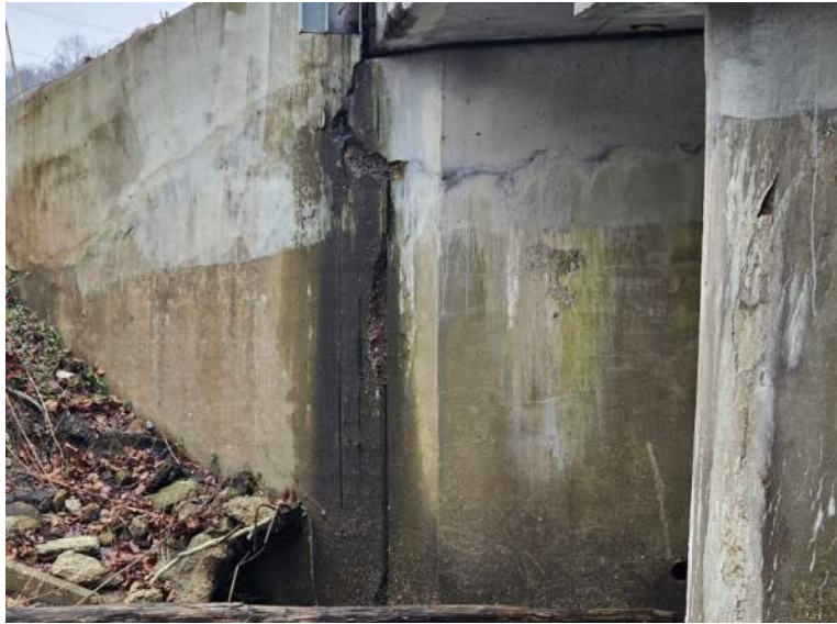
Photograph 3: Spalling on abutment
