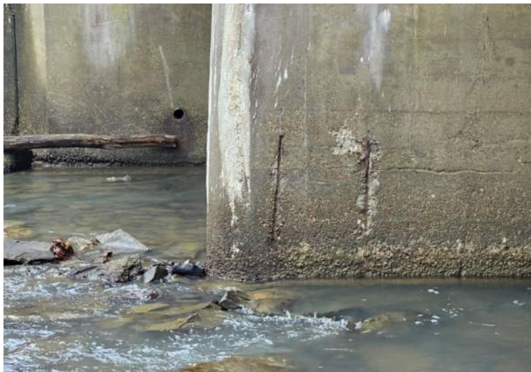
Photograph 2: Spalling and exposed reinforcing steel on pier
