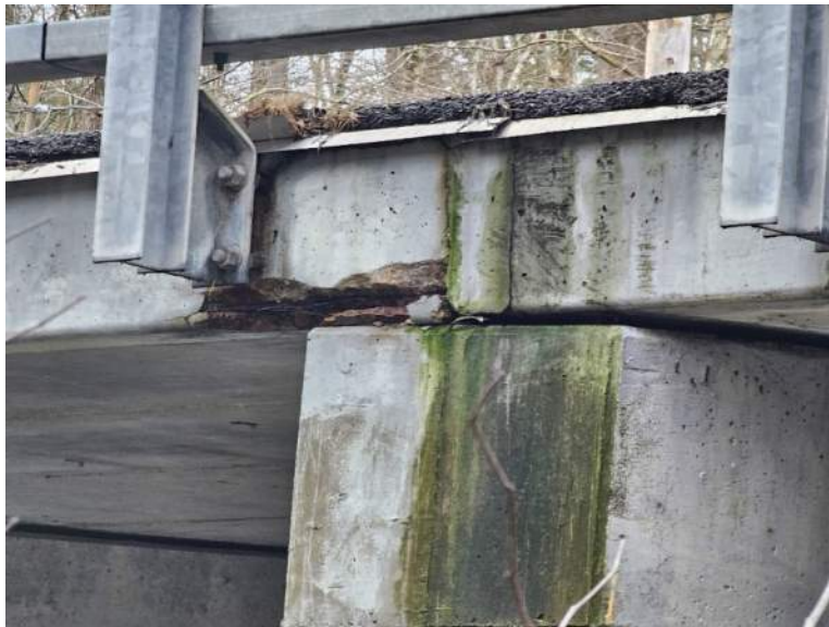
Photograph 2: Spalling and exposed steel on outer box beam
