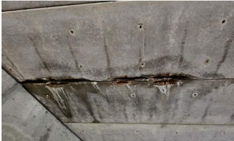
Photograph 1: Spalling and exposed steel on inner box beam
