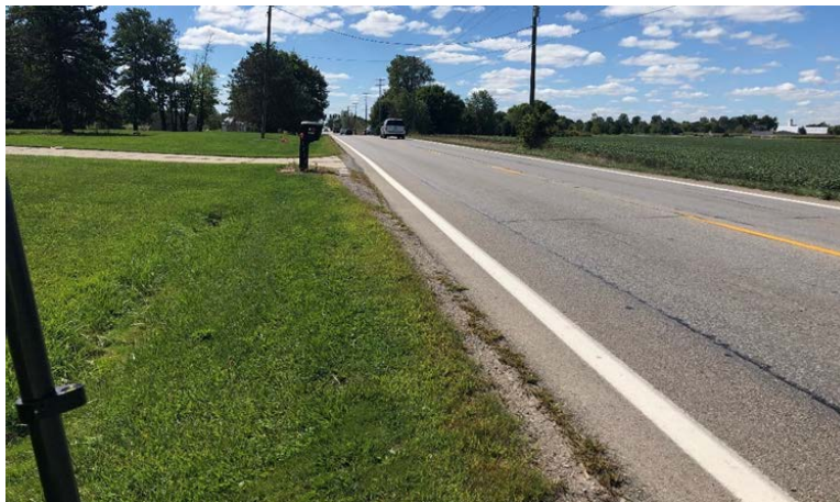
Photograph 5: Pavement condition of US-42 from Harriott Road to End
