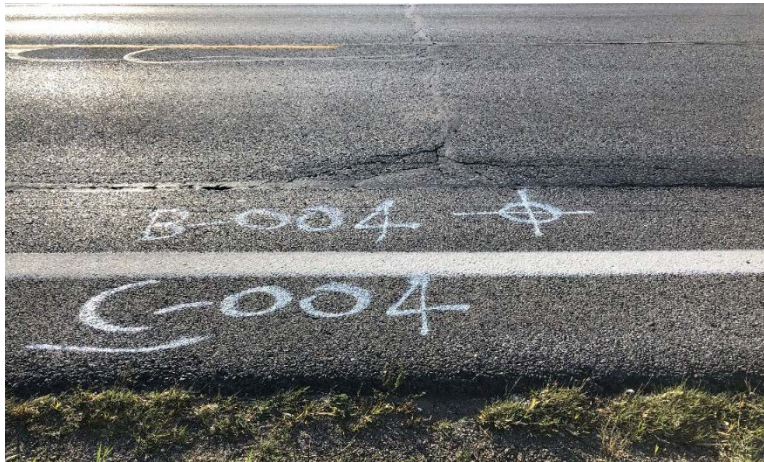
Photograph 2: Signs of standing water off eastern shoulder of US-42
