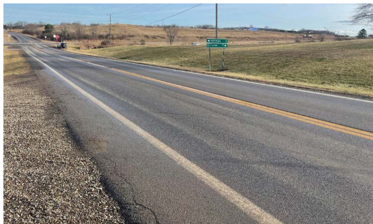
Photograph 1: Overall Pavement Condition of SR-604
