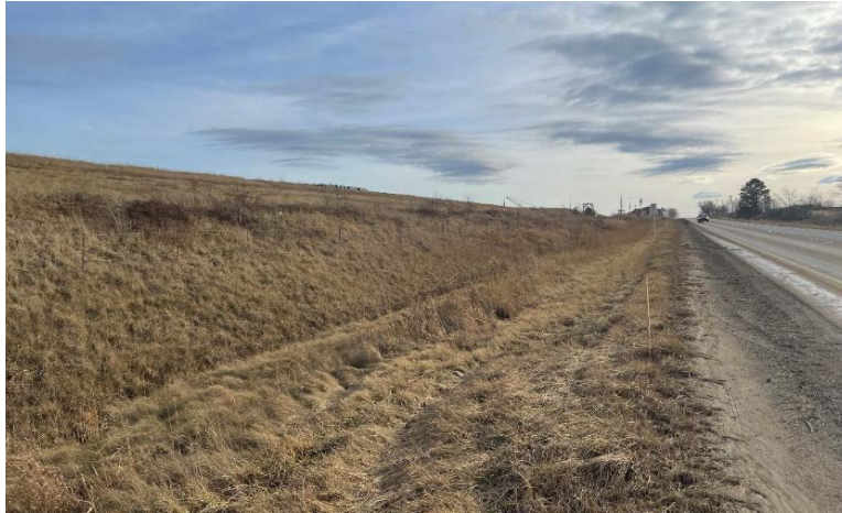
Photograph 4: Minor Signs of Standing Water in Drainage Ditch East of SR-57
