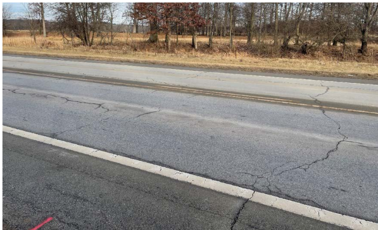
Photograph 3: Overall Pavement Condition of SR-57
