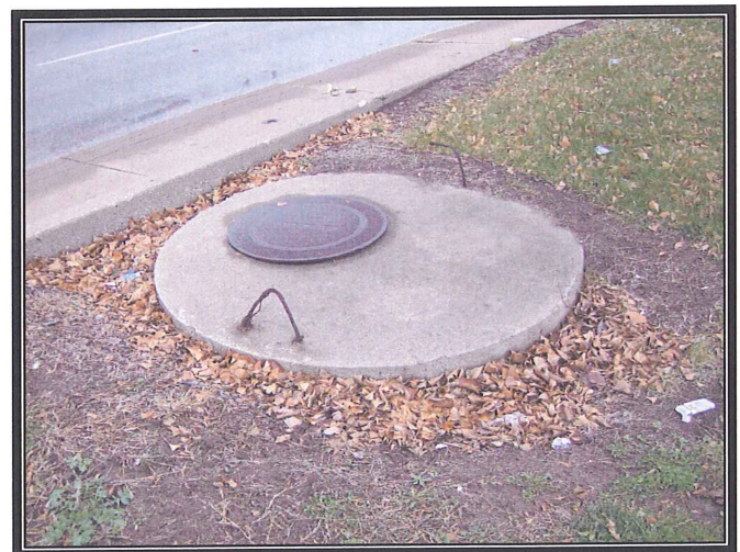
Photograph 8 View of a water meter located centrally along the northeastern border of the Property.
