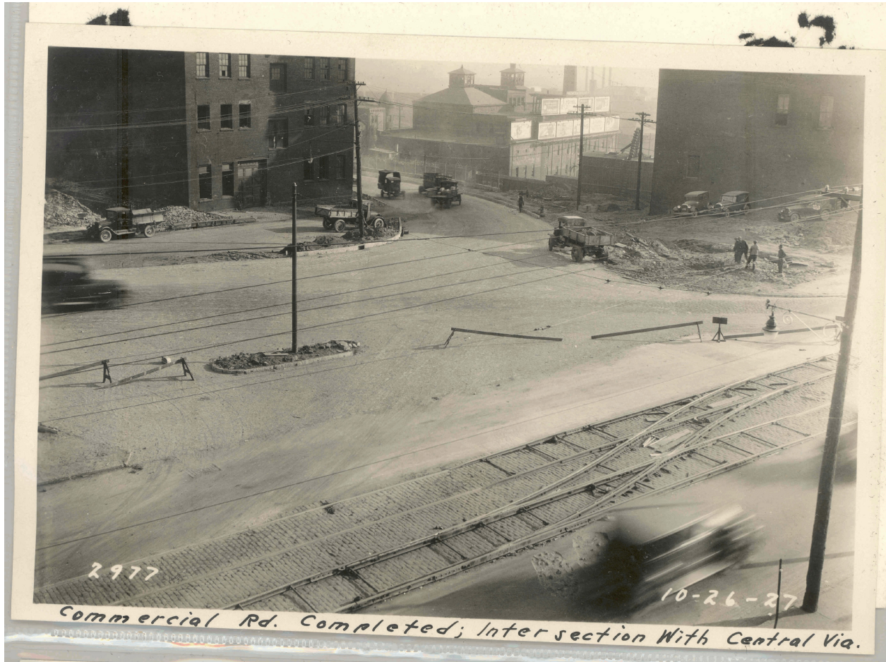
Figure 2. This October 1927 photo shows work in progress to reconfigure the intersection of Commercial Road and Central Viaduct. The Terminal Oil Company filling station would be built afterwards south of the new intersection adjacent to the Strong Cobb & Company building (right). Source: Cleveland Union Terminal Archives, Cleveland State University.
