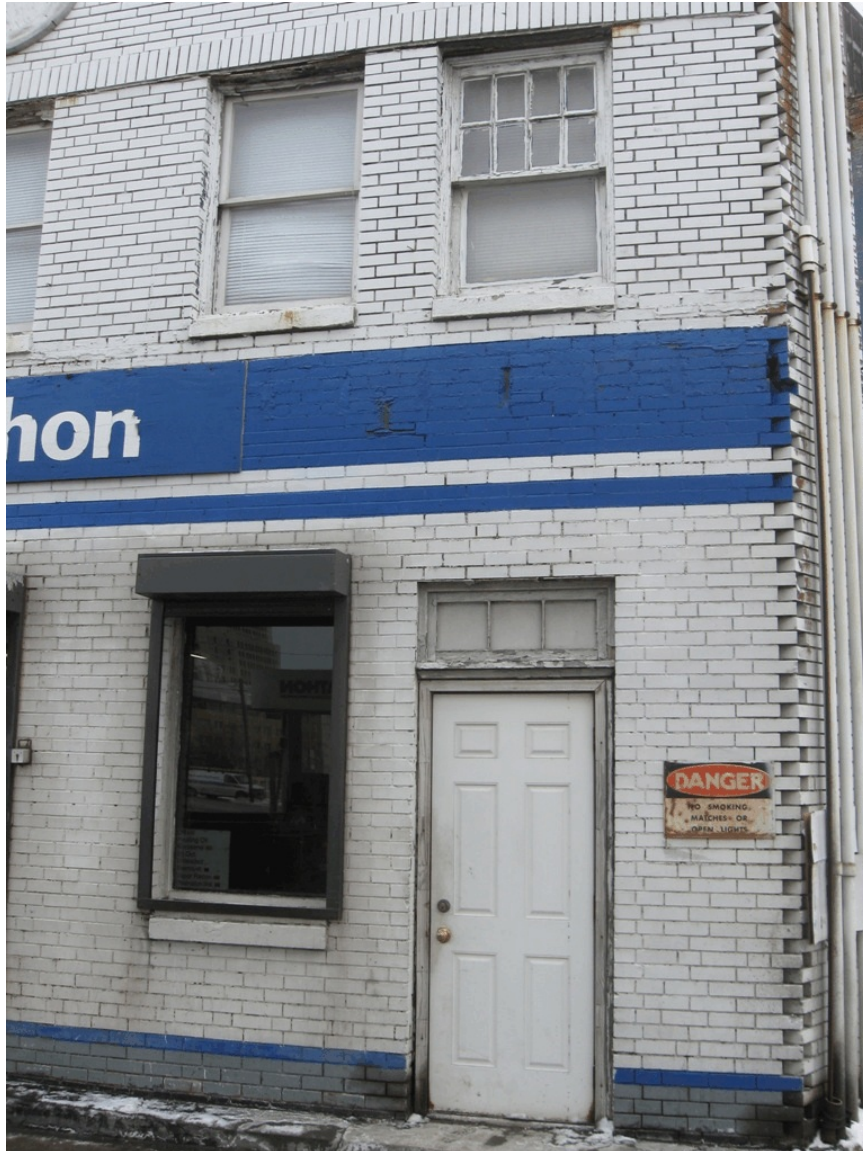
TO-6. Detail of North Elevation at West End of Building. Looking Southeast.
