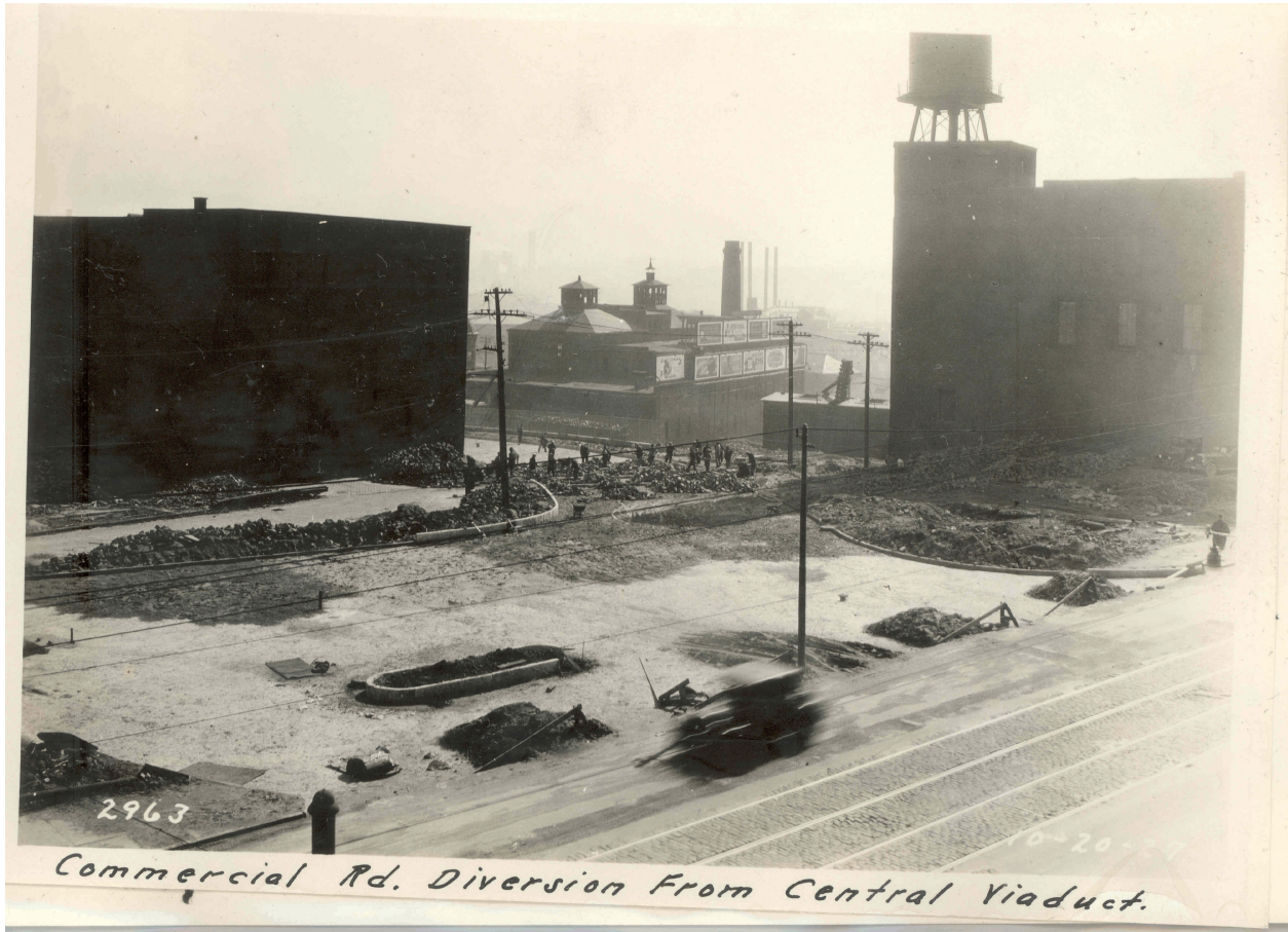
Figure 3. This October 1927 photo shows work in progress to reconfigure the intersection of Commercial Road and Central Viaduct. The Terminal Oil Company filling station would be built afterwards south of the new intersection adjacent to the Strong Cobb & Company building (right). Source: Cleveland Union Terminal Archives, Cleveland State University.
