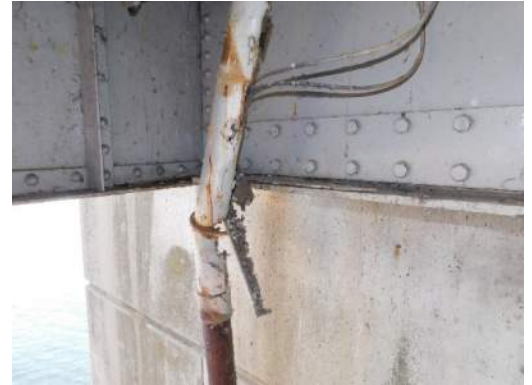
Span 6 at Pier 5, broken conduit below East sidewalk
