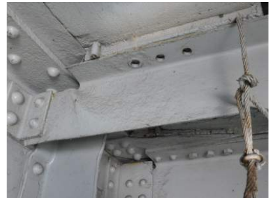
Span 4 East sidewalk support at FB35s, buckling web with pinhole
