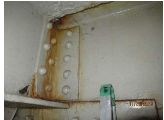
Span 10 Stringer 3W at FB11s, hole in web
