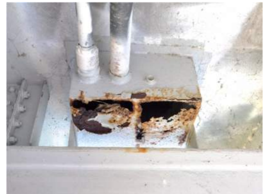
Span 3 junction box at FB18s east exterior, corrosion holes in box
