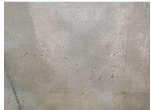
Span 2 deck underside typical shrinkage map cracking and honeycombing
