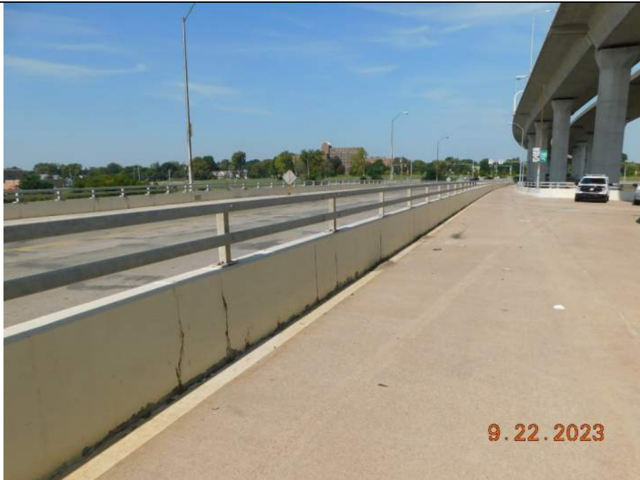
Photo S-96 - [Span 7] -East roadway / trail barrier, typical full height vertical cracking , Looking North
