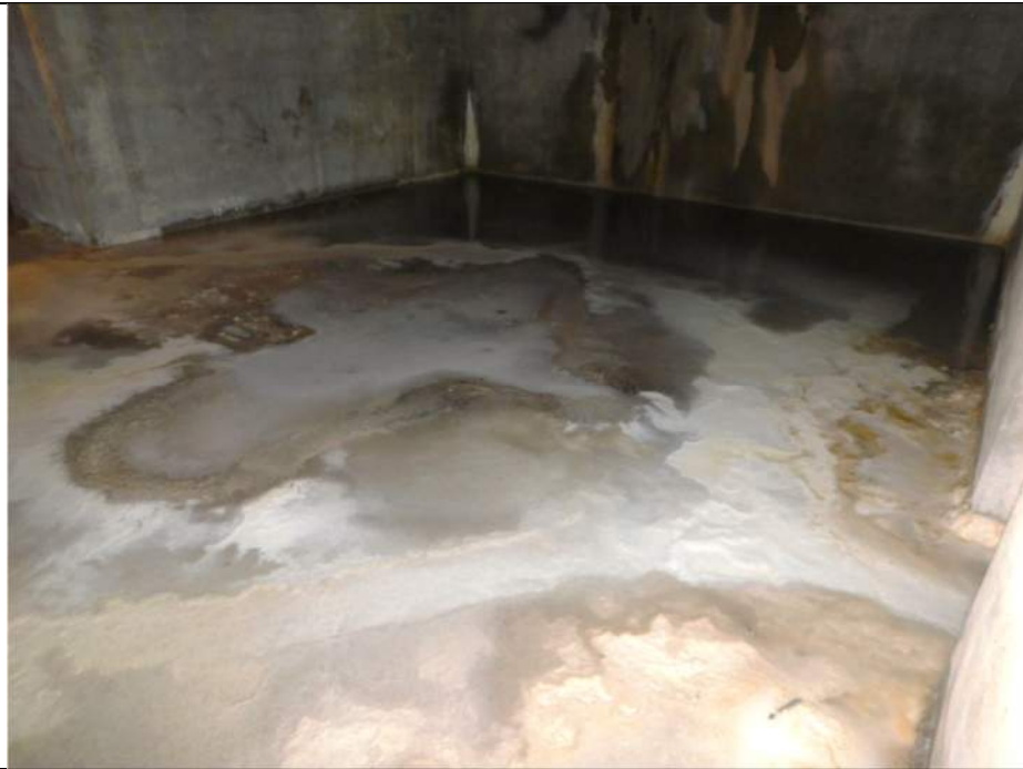
Photo S-340 - [Pier 4 Interior] -Basement Level (Level F), Room 4W, water and silt accumulation across floor, Looking South
