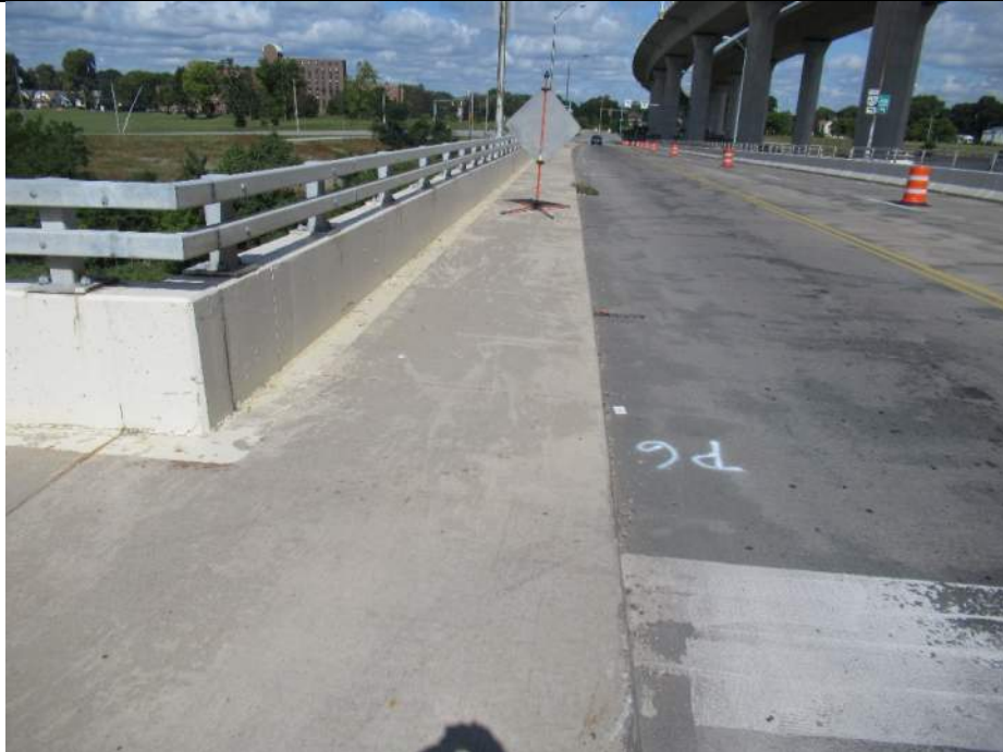
Photo S-115 - [Span 7] -West sidewalk, barrier and railing, good condition general view, Looking North
