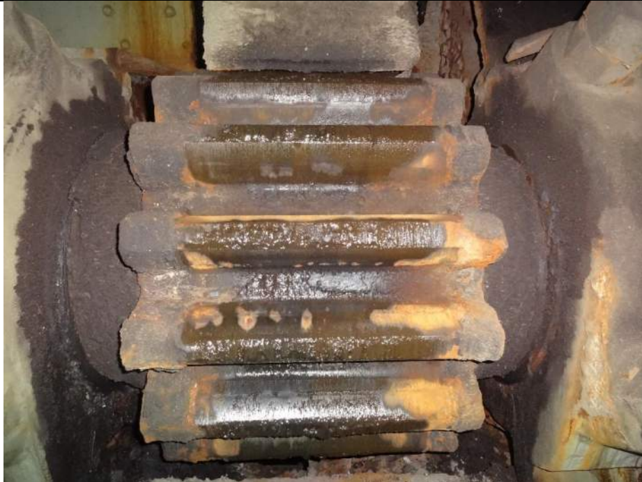
Photo 29 - [NW P1 Gear] – Note poorly lubricated P1 gear with contaminated lubrication that contains dirt and debris.
