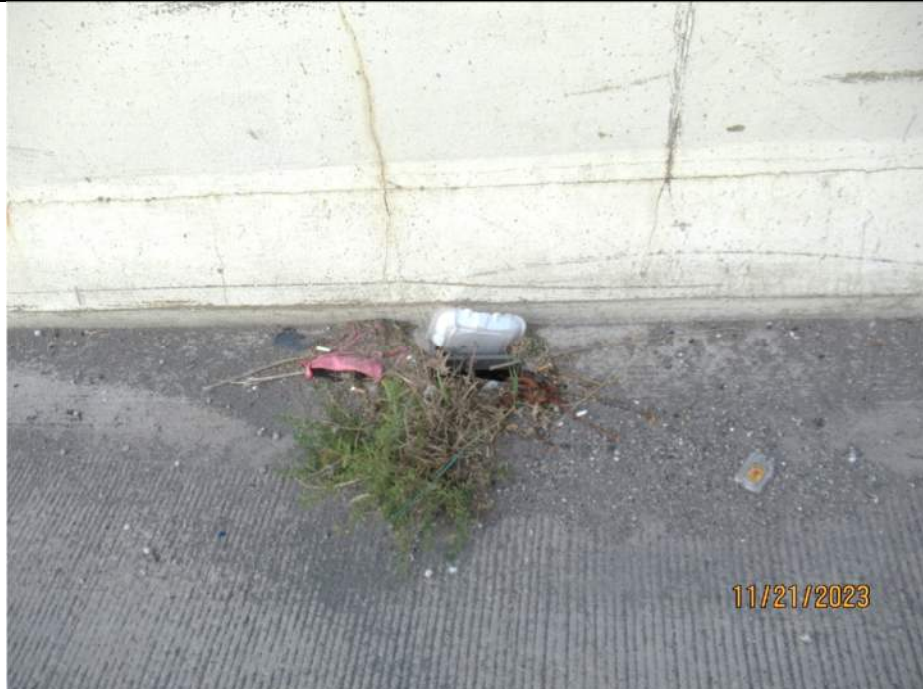
Photo S-148 - [Span 3] -Typical clogged roadway drain next to west barrier, 2nd drain south of Pier 3, Looking West
