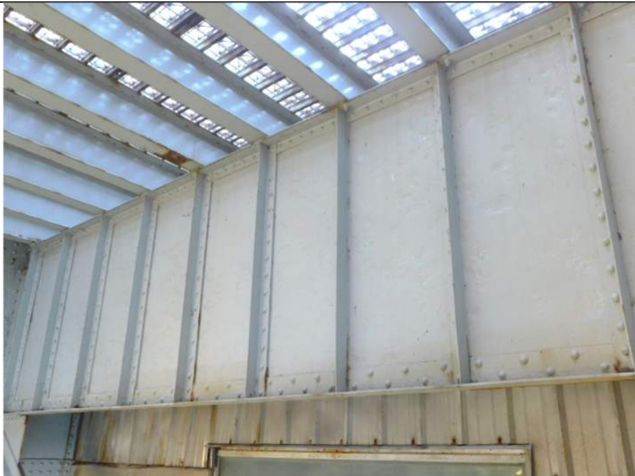
Photo S-216 - [Span 5, South Leaf] -Floorbeam 7s between G2W-G3W, typical section loss scattered throughout web, Looking South
