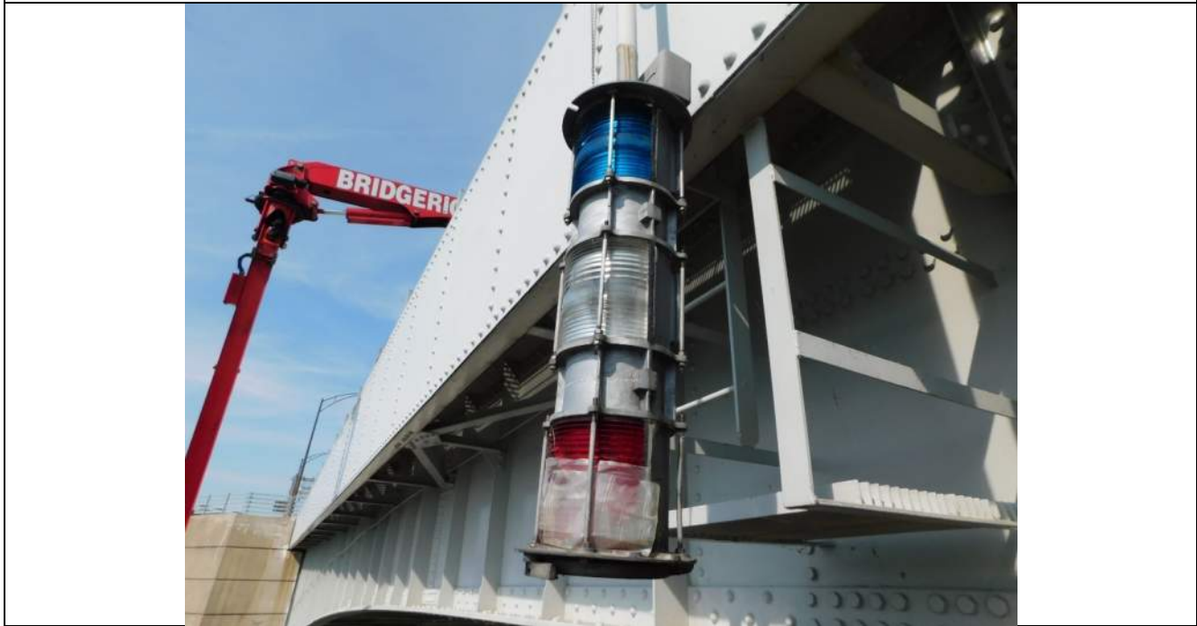
Photo S-322 - [Span 5] -West side, north navigational light, cracked glass at bottom light, lights not functional, Looking North
