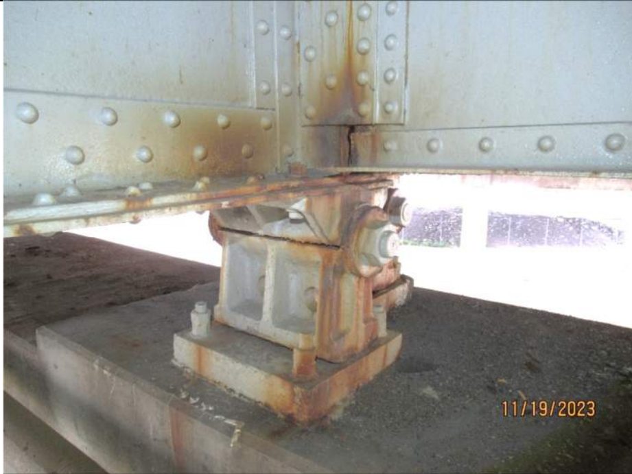
Photo S-267 - [Pier 8] -Bearing 3W (Span 9 side), moderate blistering and bleeding corrosion with staining throughout, generally plumb, Looking Southeast
