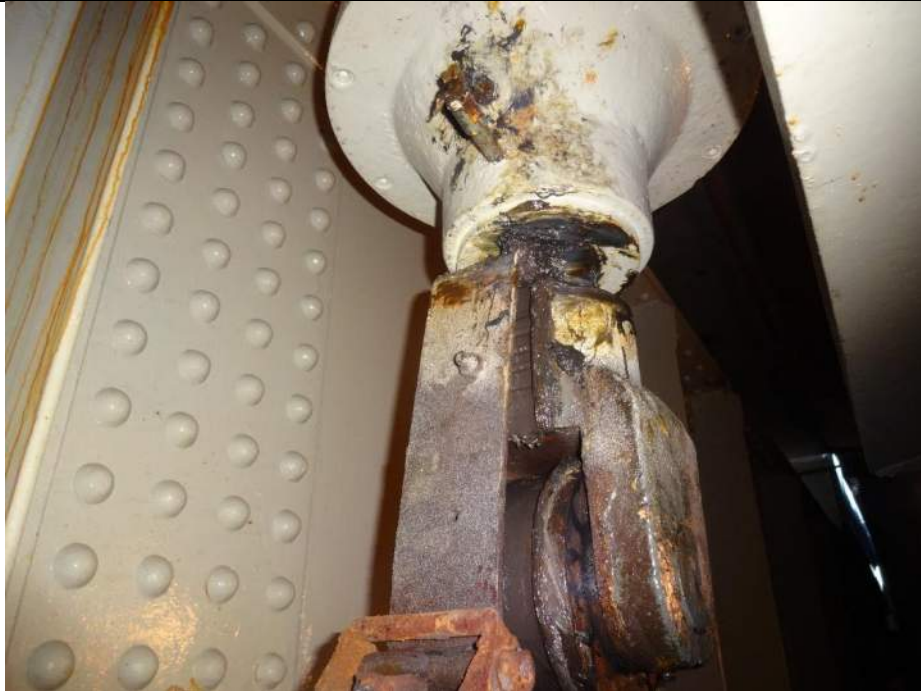
Photo 57 - [SW Seated Buffer] - Seated buffer exhibits minor surface corrosion and corrosion on back lever that is meant to extend rod.
