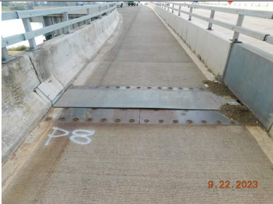
Photo S-146 - [Pier 8] -Expansion joint at East sidewalk / trail, diamond plating cover pushed upward in the middle, Looking South
