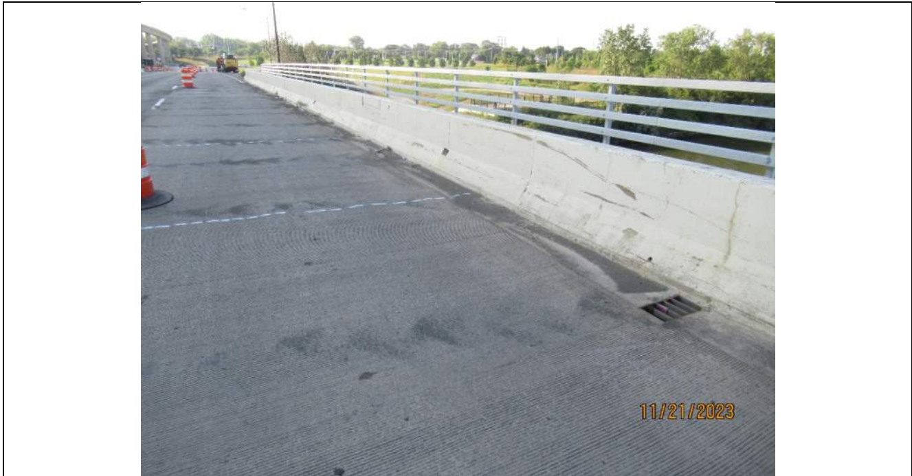
Photo S-85 - [Span 2] -West roadway barrier, typical minor impact scrapes and vertical cracking, Looking Southwest
