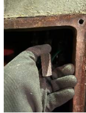
Photo E10: Southeast Main Drive Motor Brush
