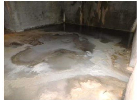
Pier 4 Basement Level F water & silt
