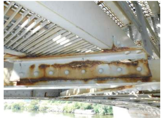
Span 5 North leaf, center catwalk support connection FB1n-FB2n with web hole
