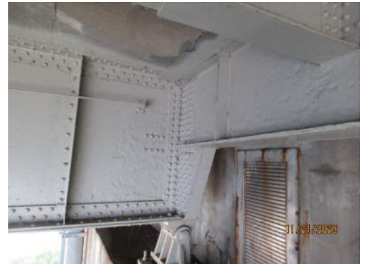
Span 9 Girder 1W bearing stiffener pack rust
