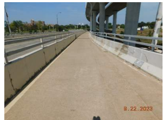
Span 8 east roadway and exterior barriers, typical cracking
