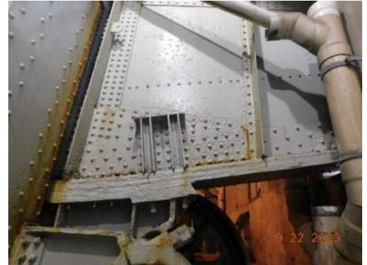
Pier 4, G3W East face widespread painted over section loss
