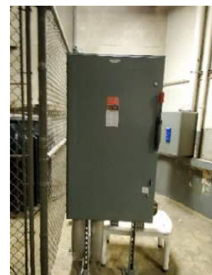
Photo E3: Service Entrance Disconnect
