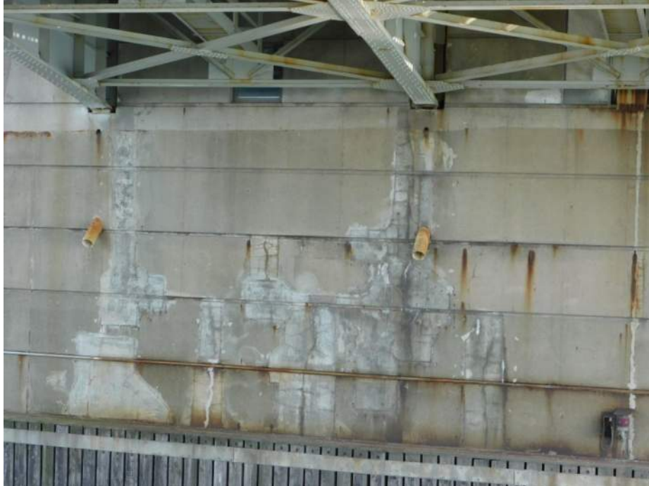
Photo S-299 - [Pier 4] -Detail view of repairs and cracking across east half of north face, Looking South
