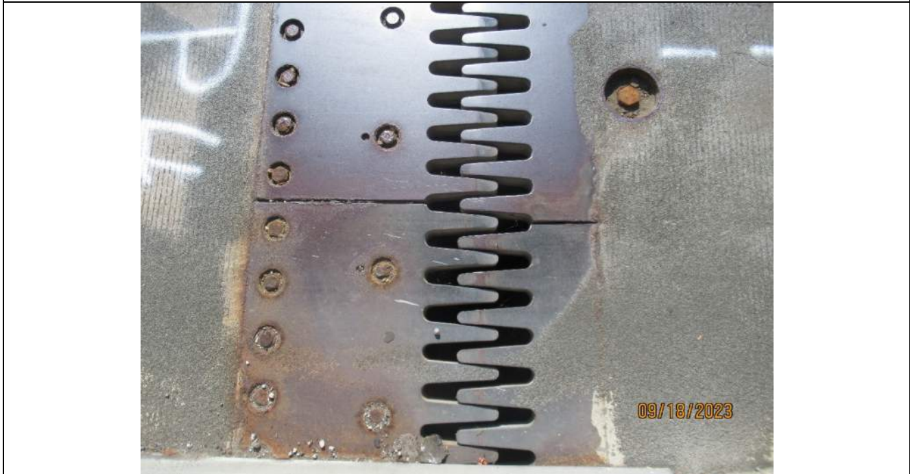
Photo S-134 - [Pier 4] -Expansion finger joint detail view at NB right lane, horizontal mis-alignment with fingers nearly touching, Looking West
