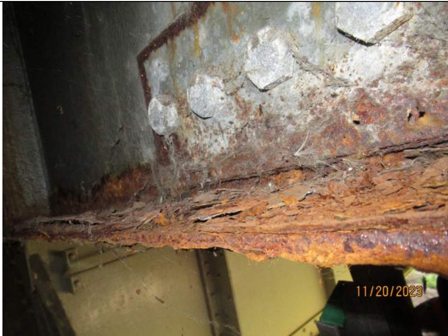
Photo S-196 - [Span 10] -Floorbeam 11S, North face bottom flange active corrosion and section loss at east half between G2W-3W, Looking East
