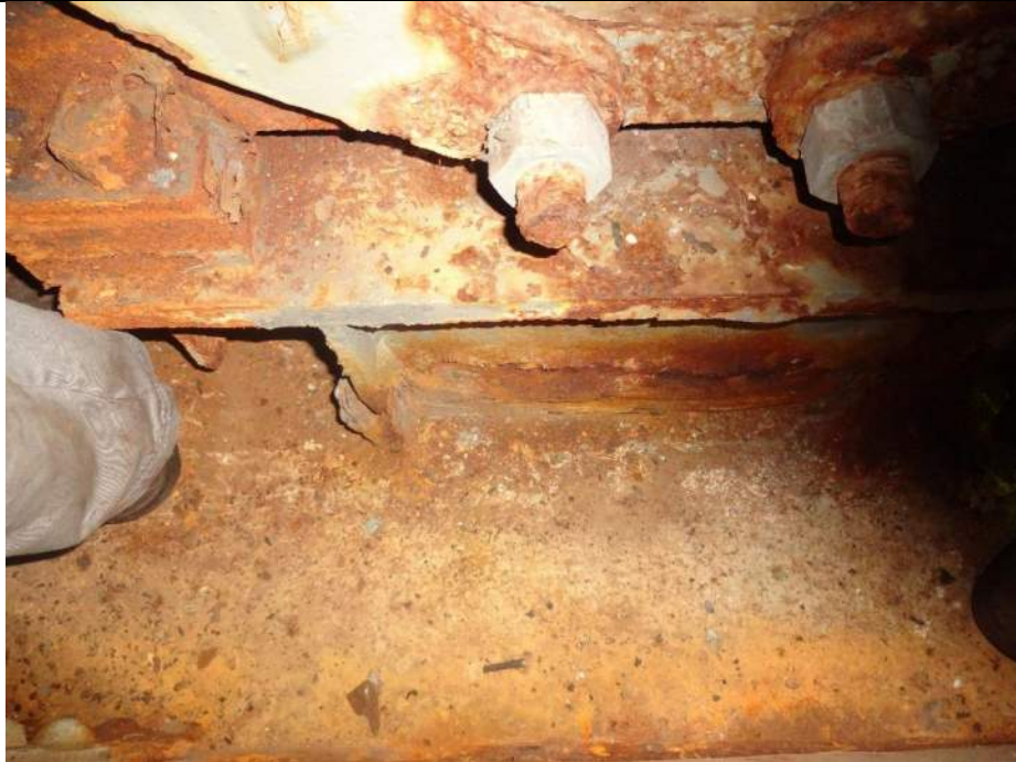
Photo 11 - [NW Motor Brake] – Note severe corrosion and section loss on motor brake support.
