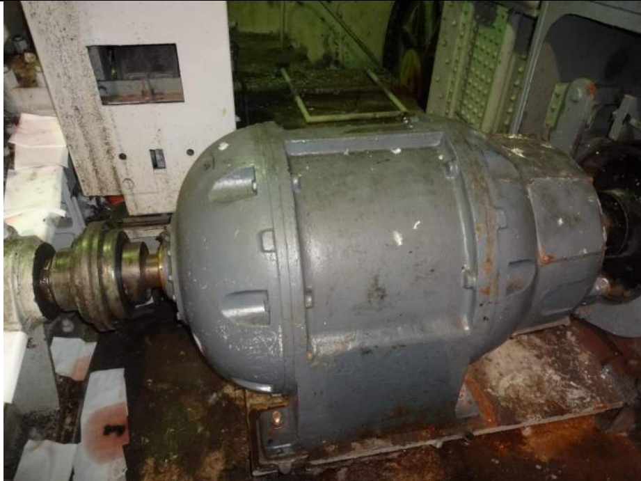
Photo 3 - [North Machinery Room] – Note surface corrosion and paint failure on motor housing and shims.
