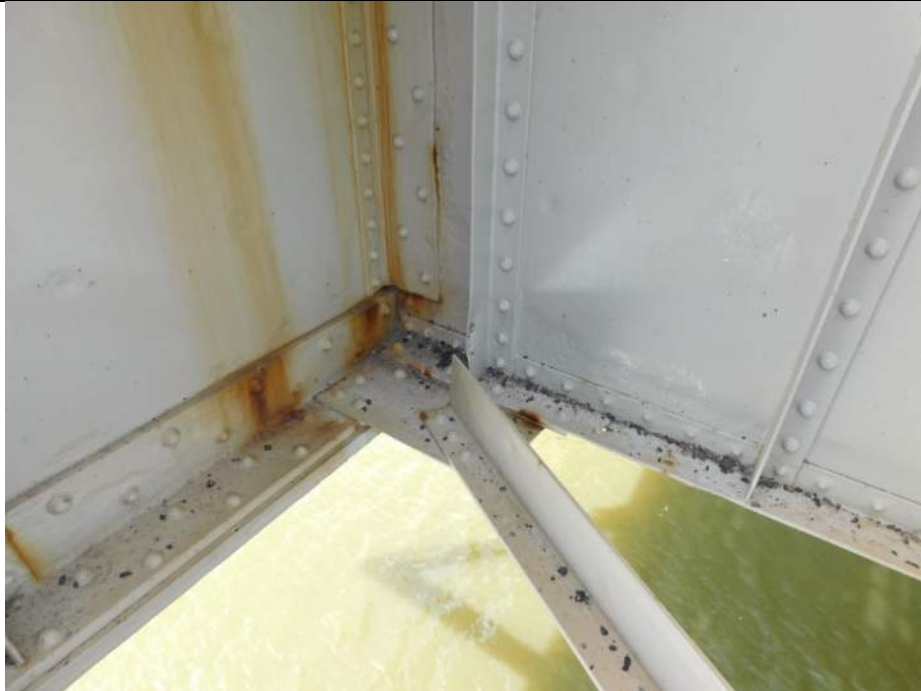
Photo S-229 - [Span 5, North Leaf] -Floorbeam 3n at east side G2W, typical section loss, minor debris, and small holes at base of web stiffener, Looking North
