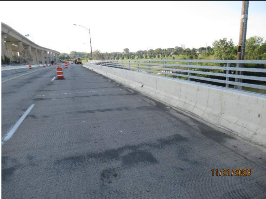
Photo S-40 - [Span 2] -Roadway deck and wearing surface, SB lanes near north end of span, Looking South
