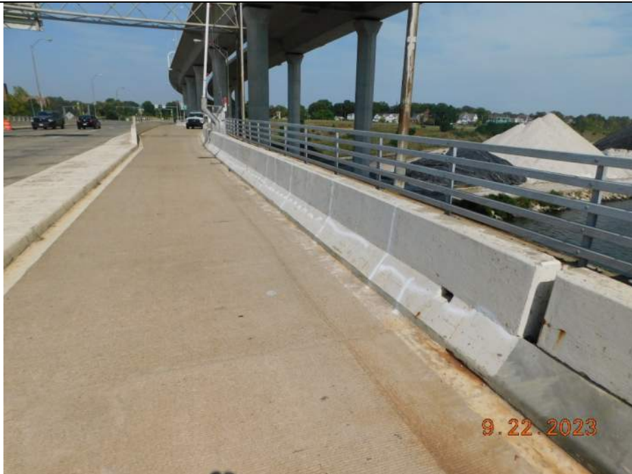
Photo S-94 - [Span 6] -East roadway / trail barrier, typical full height vertical cracking and isolated longitudinal cracking at lower slope, Looking North
