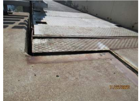
Span 5 North leaf East sidewalk at rear break
