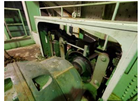
Photo E11: Northeast Motor Brake
