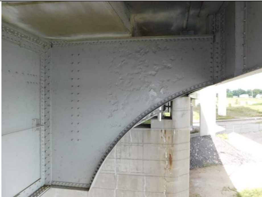
Photo S-200 - [Span 6] -Floorbeam 6S, East exterior, South face, typical painted over section loss up to 0.125" deep across the east half of the web, Looking North
