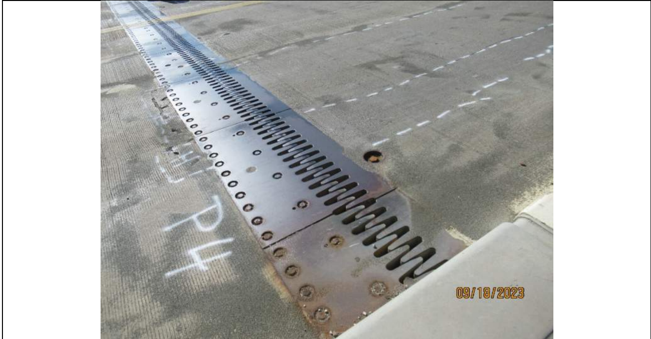
Photo S-133 - [Pier 4] -Expansion finger joint general view across NB roadway lanes, Looking Northwest
