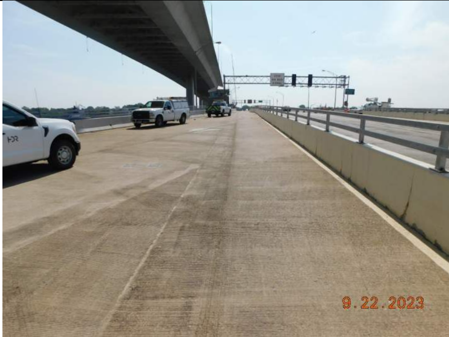
Photo S-63 - [Span 7] -Roadway deck and wearing surface, East trail and flare area, Looking South
