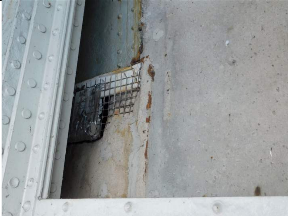
Photo S-297 - [Pier 4] -Hole in pier wall with temporary repair, south wall of pier at Girder 3W, Looking North
