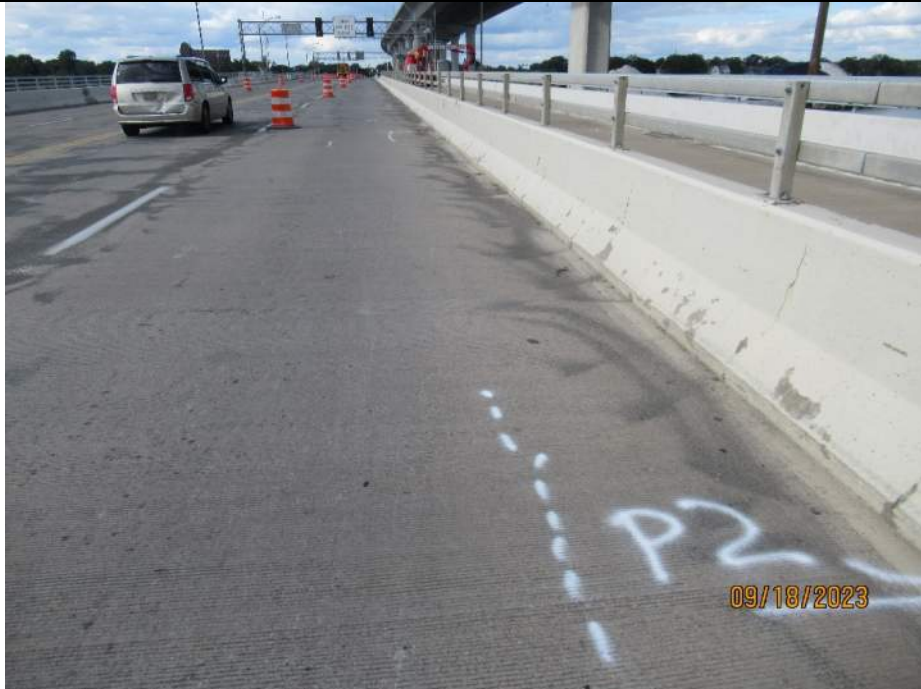
Photo S-42 - [Span 3] -Roadway deck and wearing surface, NB lanes at south end of span, Looking North
