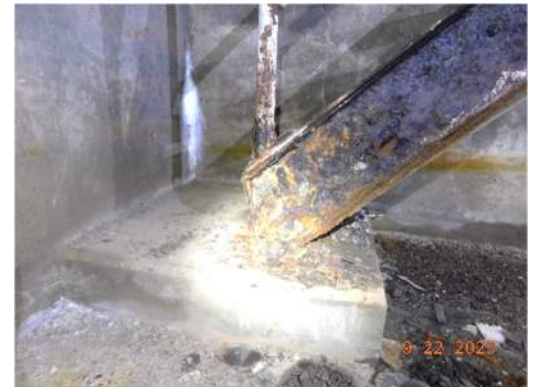
Pier 5 base of stairs at Level F heavy corrosion and hole in web
