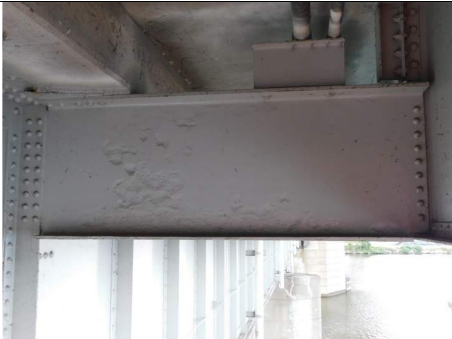
Photo S-198 - [Span 3] -Floorbeam 20S, East exterior, South face, typical painted over section loss up to 0.125" deep across lower web, additional similar loss in middle web, Looking North
