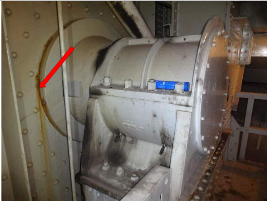
Photo 36 - [SW Inner Trunnion] - Corrosion is present on collars of trunnion bearings.
