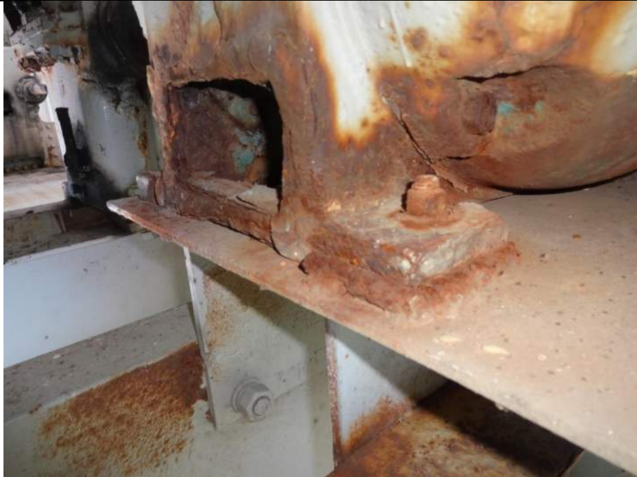
Photo 41 - [Span Lock Motor ] – Note heavy corrosion on SE motor foot mount.
