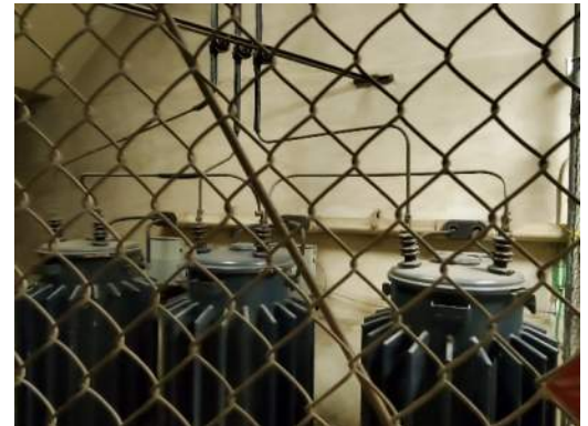
Photo E2: Medium Voltage Transformers in the Control House
