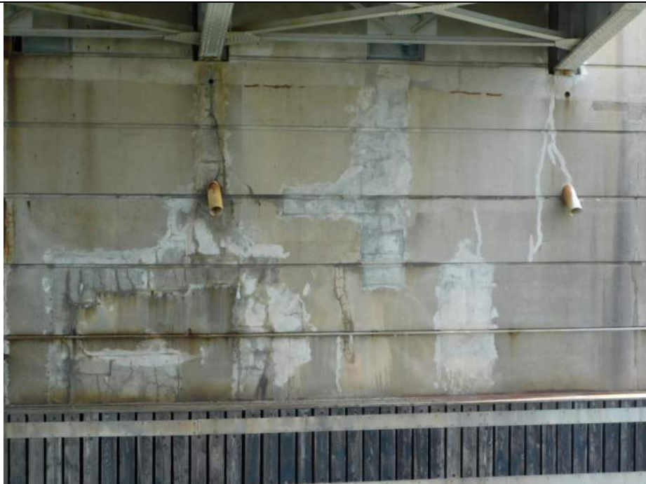
Photo S-298 - [Pier 4] -Detail view of repairs and cracking across west half of north face, Looking South
