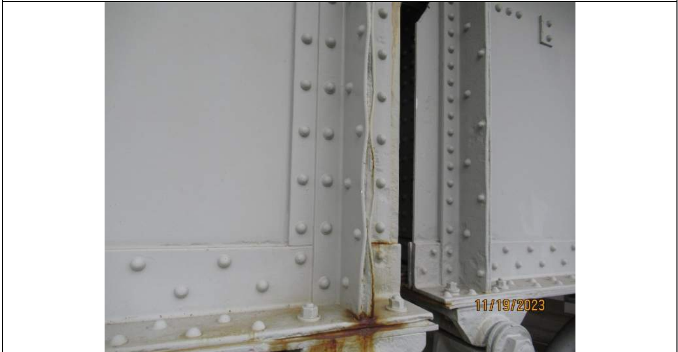
Photo S-184 - [Span 9] -Girder 1W west bearing stiffener angles at Pier 8 exhibit up to 1.25" thick packing corrosion and warping between the outstanding legs, Looking East
