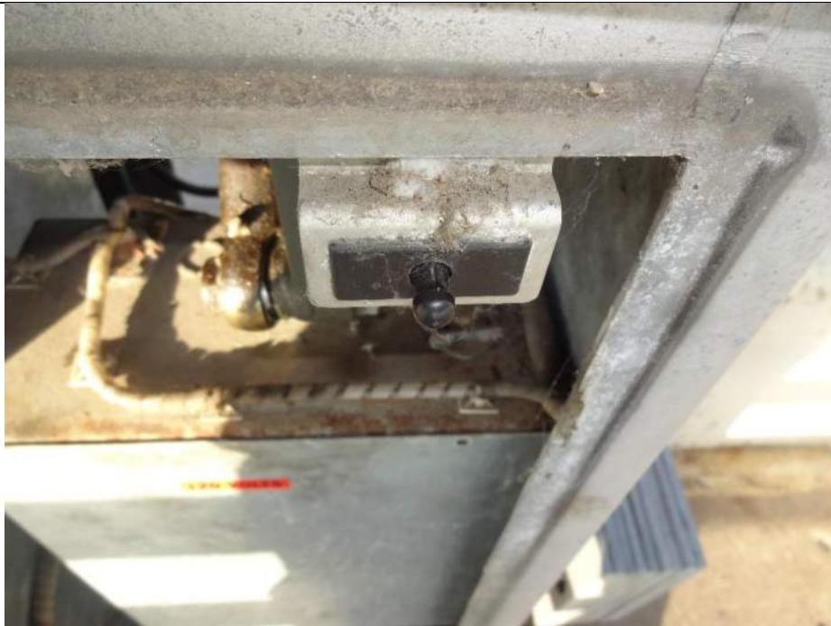
Photo 68 - [NE Traffic Gate] - East door limit switch on vertical arm traffic gate does not extend.
