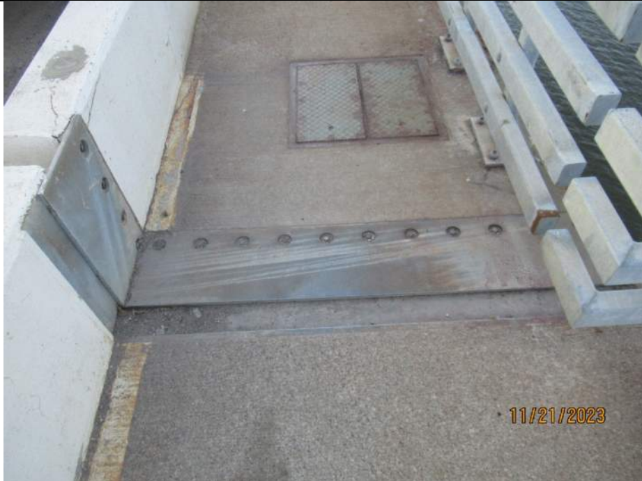
Photo S-137 - [Pier 5] -West sidewalk expansion joint with minor debris, general view, Looking South
