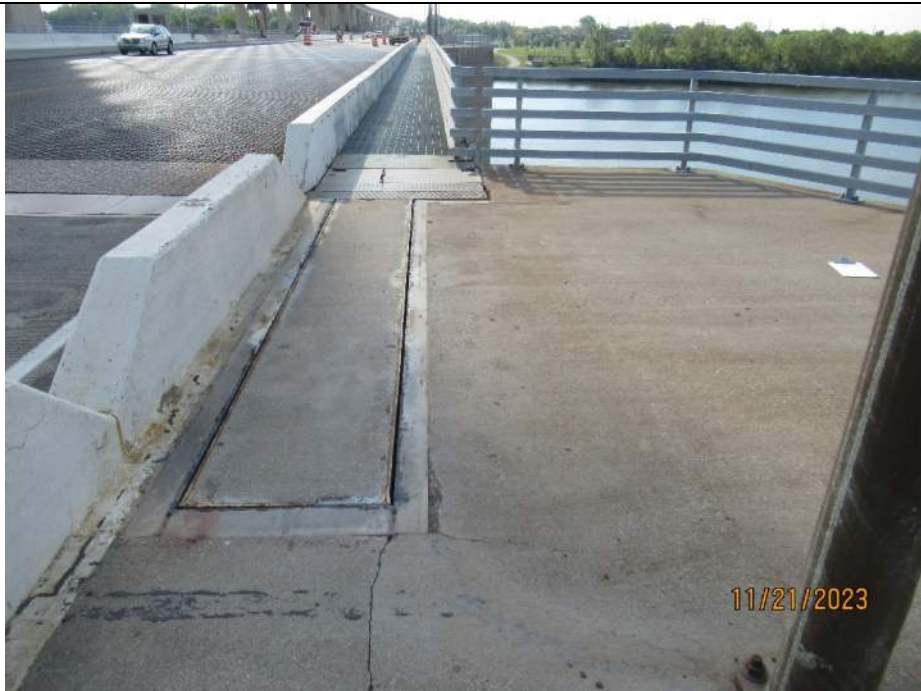
Photo S-112 - [Pier 5 Span] -West sidewalk and railings, good condition general view, Looking South
