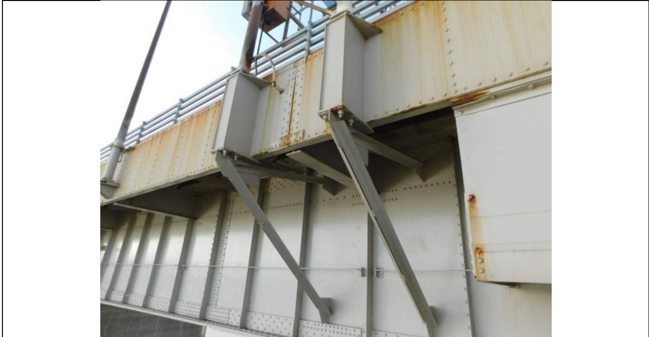
Photo S-325 - [Span 4] -Overhead Sign Gantry, general view of east side support framing / attachment to fascia and G4W, Looking Southwest
