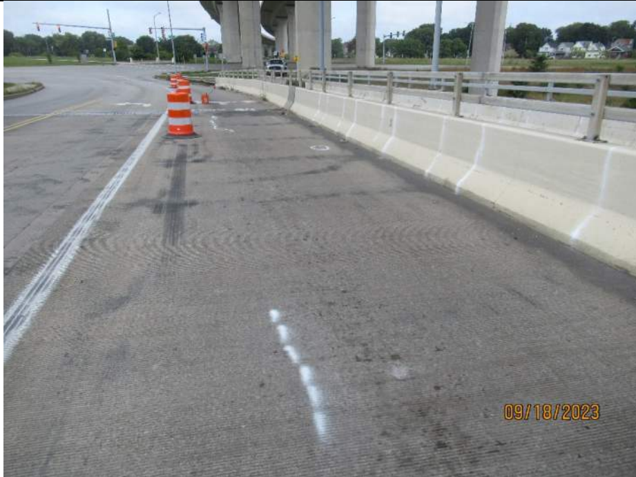
Photo S-67 - [Span 10] -Roadway deck and wearing surface, NB right lane from midspan, Looking North
