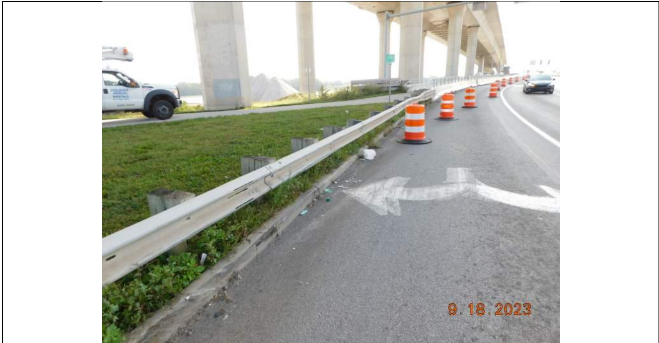
Photo S-27 - [North Approach] -Northeast guard railing approach, minor impact damage, Looking Southeast
