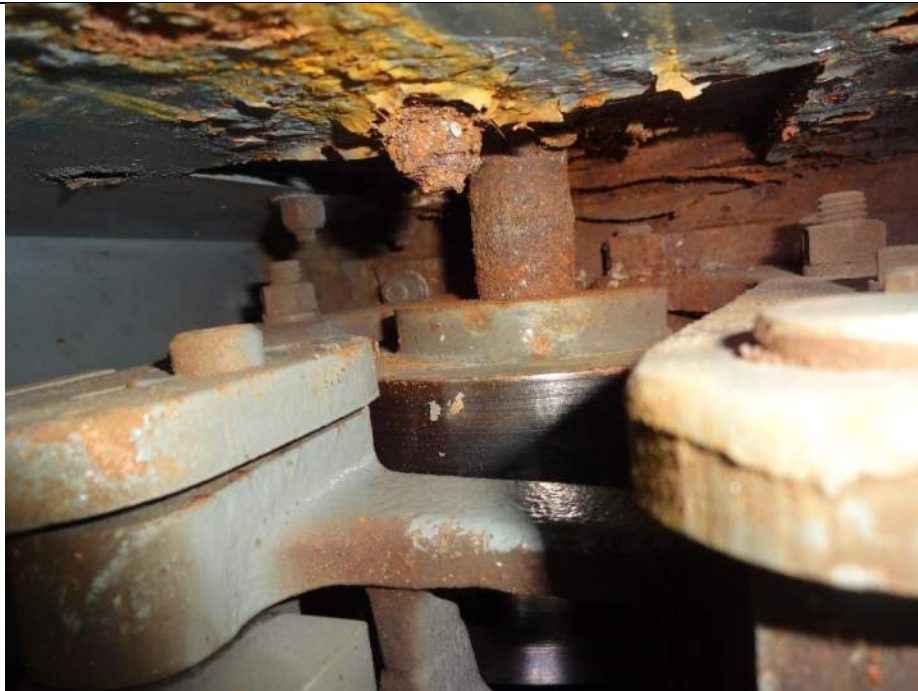
Photo 38 - [Span Lock Thruster Brake] – Note severely corroded thruster brake shaft on span lock. Linkages are also not well lubricated.
