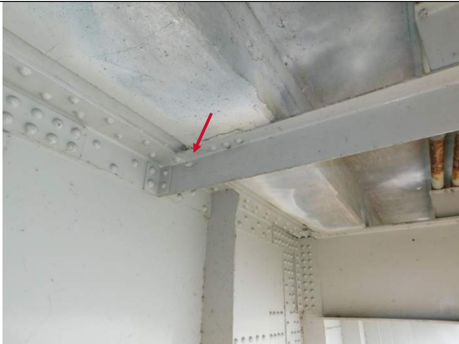
Photo S-204 - [Span 4] -Sidewalk framing member with section loss and a 2" diameter hole in the web below deck curb location, between Floorbeams 35S-36S at west sidewalk, Looking Southeast
