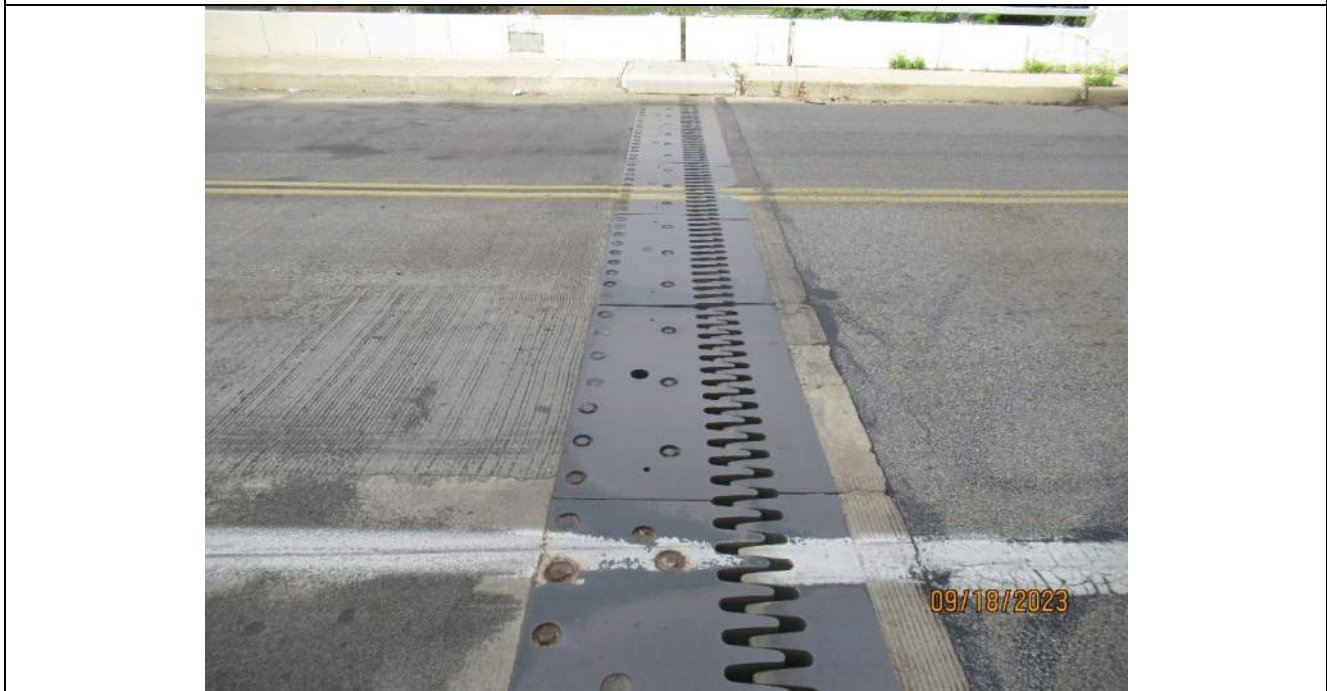
Photo S-130 - [North Abutment] -Abutment reference line finger joint at NB left lane and SB lane, Looking West
