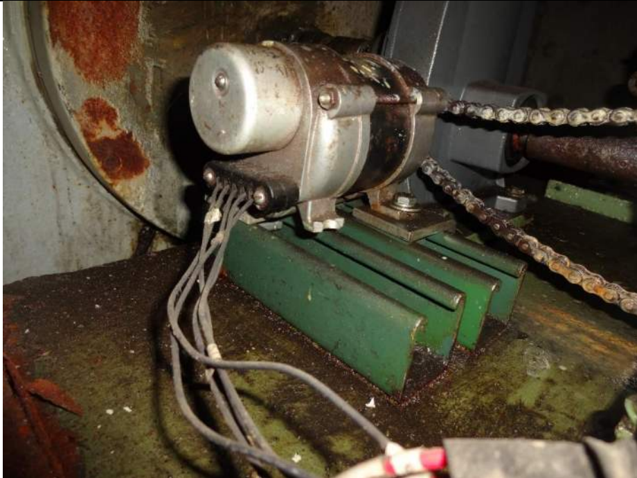
Photo 33 - [South Machinery Room] - South side span drive control machinery has missing foot mount on selsyn motor and a loose chain.
