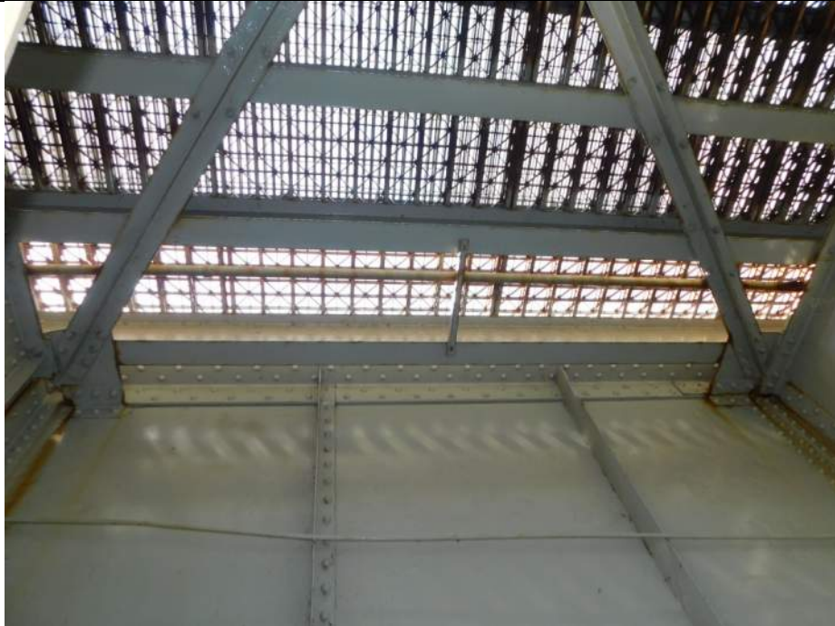
Photo S-333 - [Span 5] -Abandoned conduit along east side of G3W between FB3n-FB4n, above floorbeam top flanges, general view, Looking West
