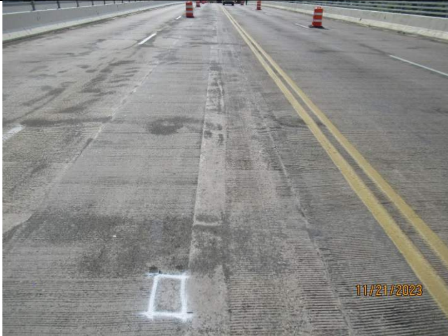
Photo S-45 - [Span 4] -Roadway deck and wearing surface, middle lanes near mid-span, Looking South
