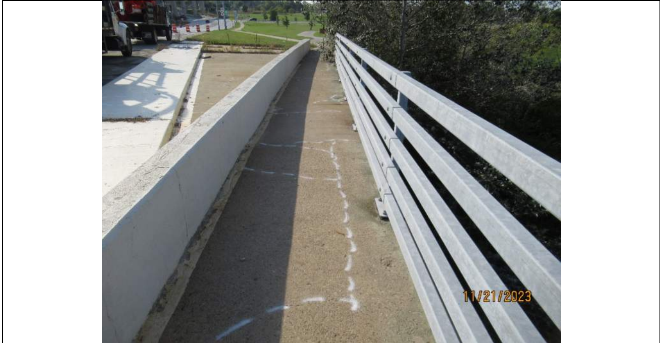
Photo S-19 - [South Approach] -Southwest sidewalk, barrier and pedestrian railing, Looking South
