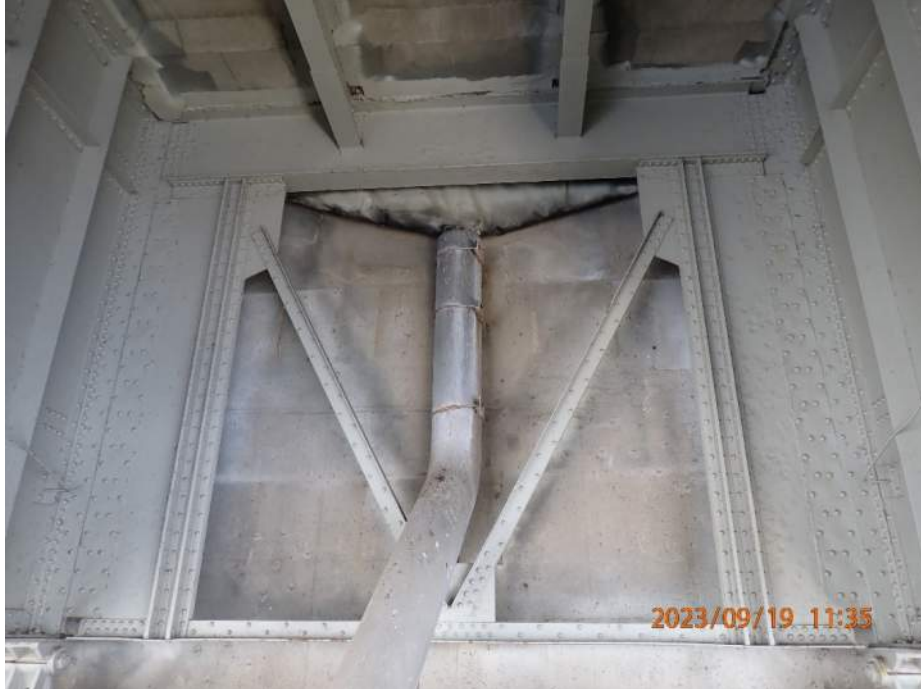
Photo S-135 - [Pier 4] -Underside of finger joint, view of elastomeric trough and drainage downspout (b/w G2-G3), connection to pier, generally good condition, Looking North
