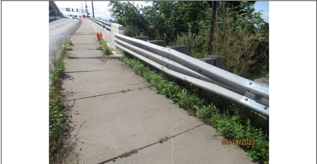
Photo S-24 - [North Approach] -Northwest guard railing transition and barrier, Looking Southwest
