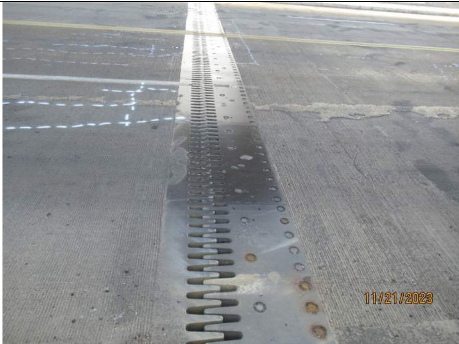
Photo S-136 - [Pier 5] -Expansion finger joint general view across SB roadway lanes, Looking East
