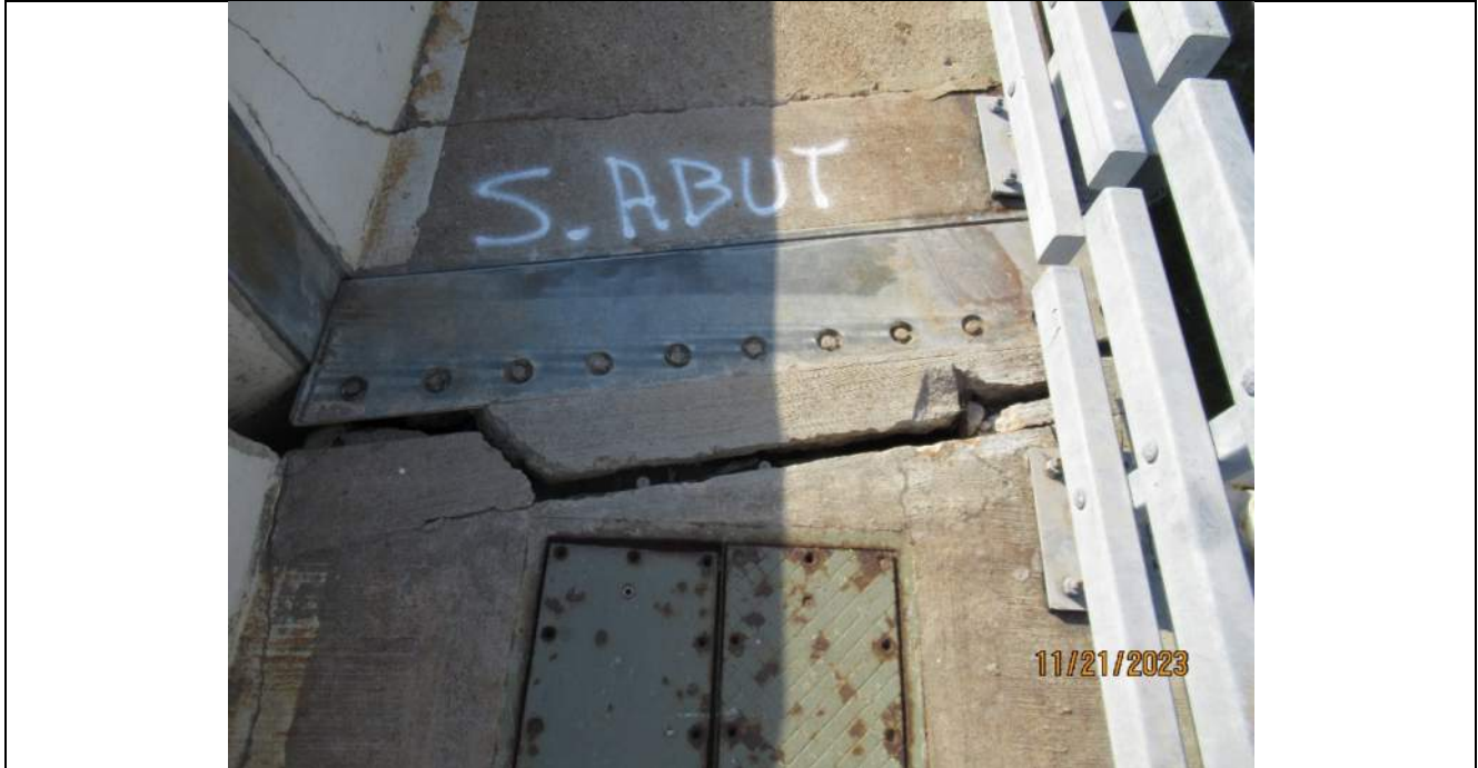
Photo S-123 - [South Abutment] -Abutment reference line sliding plate joint at West sidewalk, joint has seized and broken apart at the north header, Looking South
