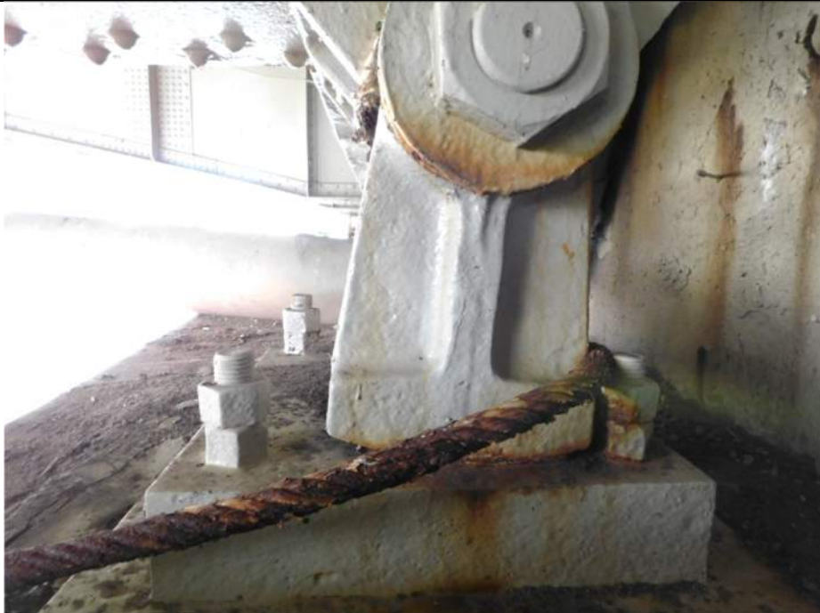
Photo S-260 - [Pier 5] -Bearing 2W at North side of Bascule Pier 5, general view of bearing tilted South in expansion, Looking West
