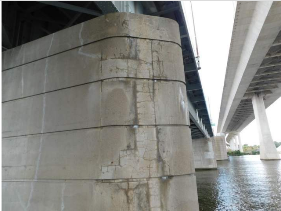
Photo S-292 - [Pier 3] -Pier south side at east end, detail view of shrinkage cracking and dampness throughout repair areas, Looking North
