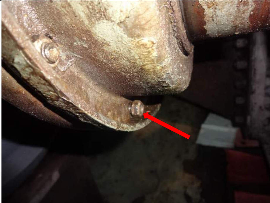
Photo 15 - [NE Coupling] – Note loose nut on coupling.
