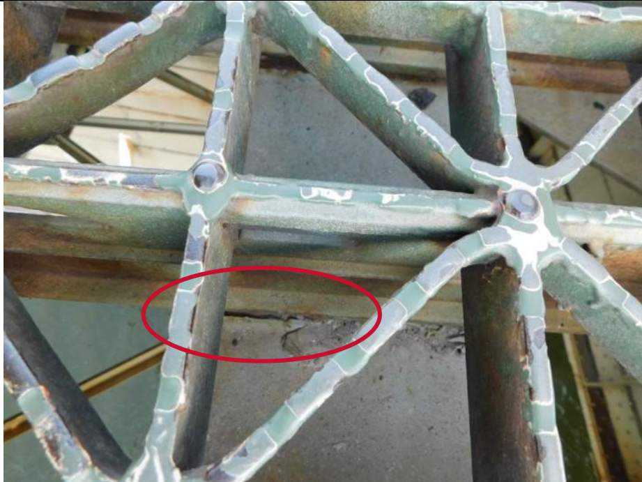
Photo S-53 - [Span 5] -Detail view of grid deck with broken weld connecting lower main bar to stringer top flange, South leaf in SB lanes near Pier 4, Looking North
