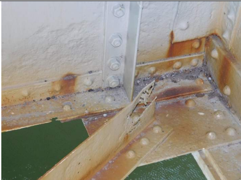
Photo S-222 - [Span 5, South Leaf] -Floorbeam 3s, north BF with 1" dia hole next to bracing connection at G3W, note 100% SL at end of bracing member, Looking Southeast
