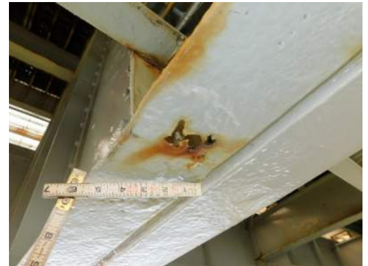
Span 5 South leaf, FB3s b/w G3W-G4W, BF hole below catwalk
