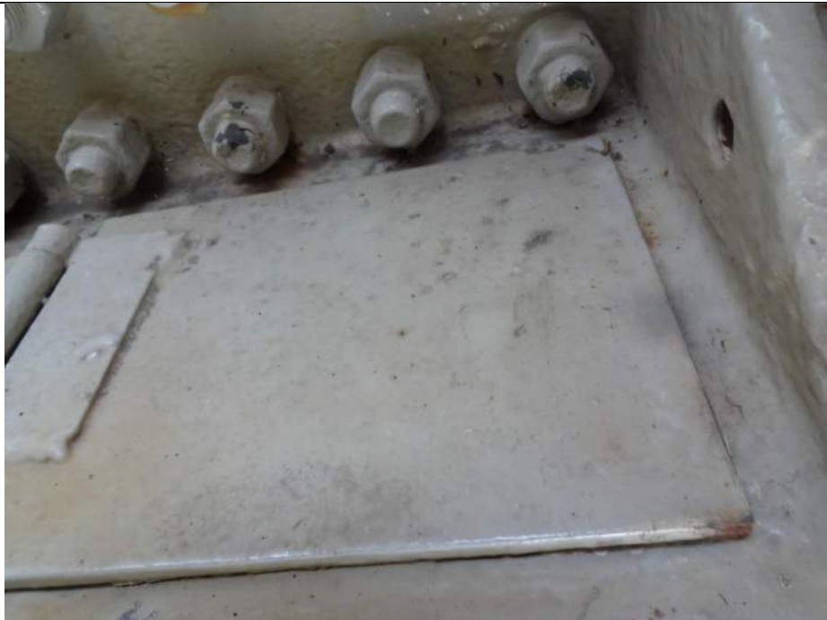
Photo 52 - [NE Outboard Locking Mechanism] - Top cover is seized due to paint.
