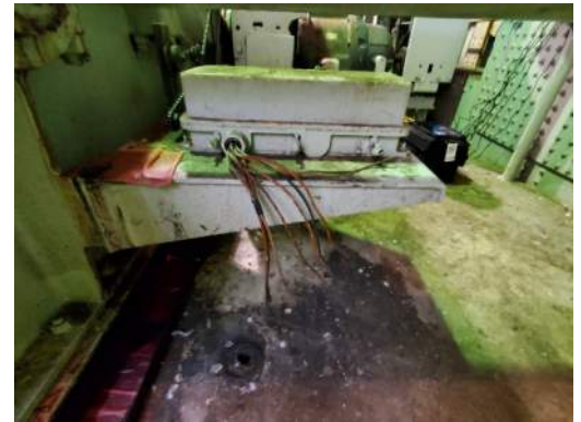
Photo E19: Abandoned Rotary Cam Limit Switch
