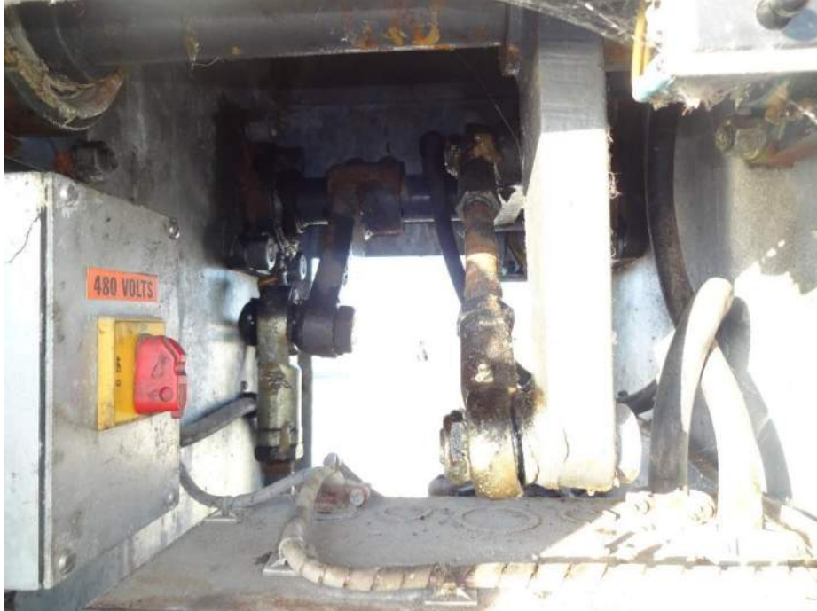
Photo 67 - [NE Traffic Gate] - Crank arm has misalignment possibly due to deformation.
