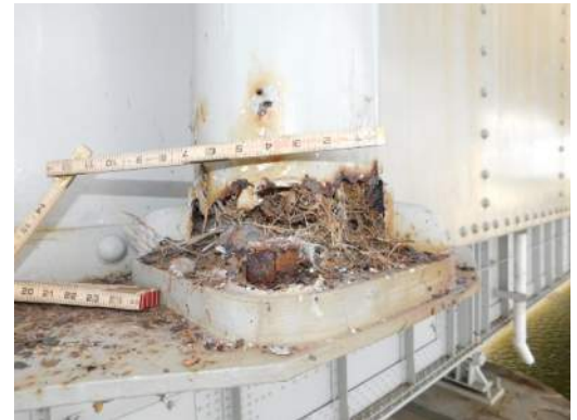
Span 3, FB25s East side light pole base with holes
