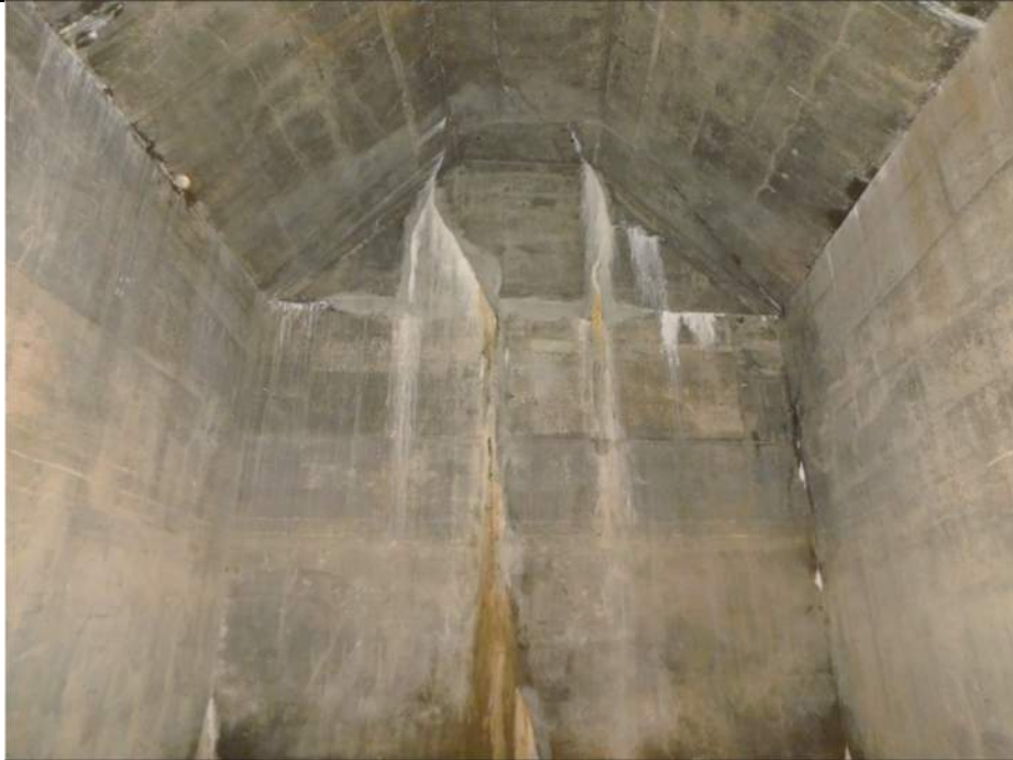
Photo S-341 - [Pier 4 Interior] -Basement Level (Level F), Room 2W, vertical cracking in North wall with heavy efflorescence, Looking North
