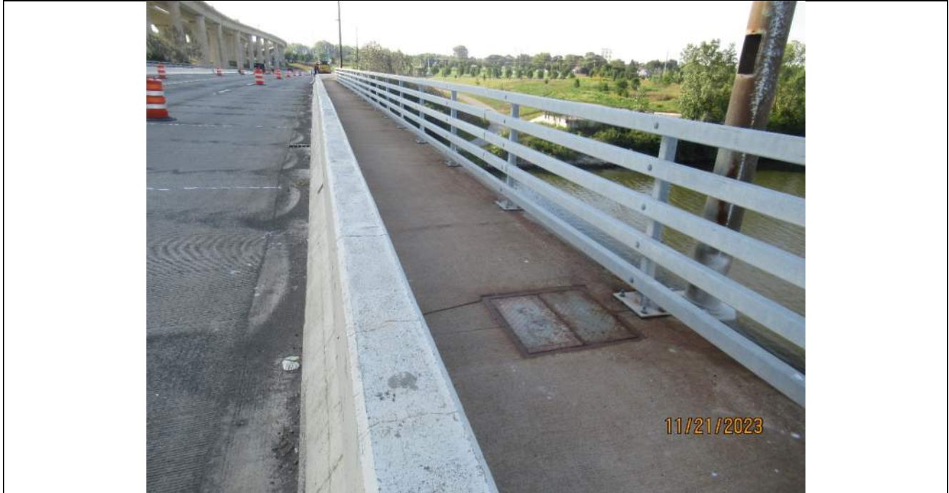
Photo S-103 - [Span 2] -West pedestrian railing and sidewalk, typical good condition, Looking Southwest
