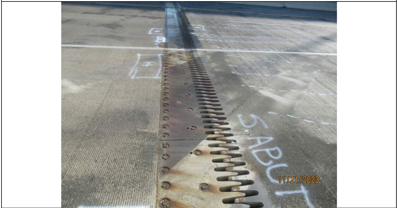
Photo S-124 - [South Abutment] -Abutment reference line finger joint general view in SB shoulder, Looking East
