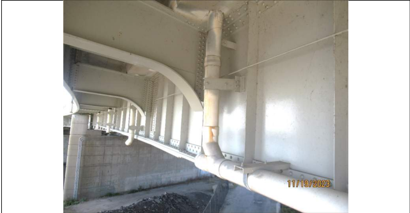
Photo S-151 - [Span 7] -Drainage downspouts, piping and supports along Girder 5W (west flare exterior girder), generally good condition, Looking Southwest
