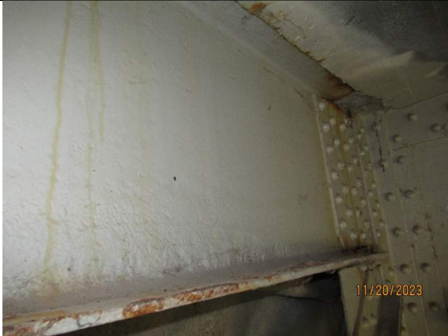
Photo S-195 - [Span 10] -Floorbeam 11S, South face east half between G2W-3W, typical section loss throughout web, Looking North
