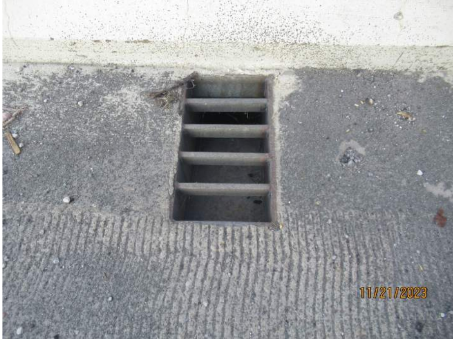
Photo S-149 - [Span 4] -Typical roadway drain next to barrier, clear and good condition, SB lanes near mid-span shown, Looking West
