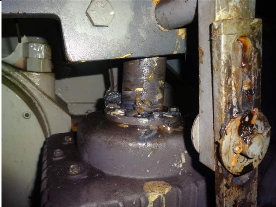
Photo 7 - [North Machinery Room] – Note oil purge from top of thruster on motor brake.
