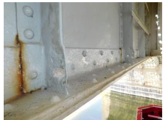
Span 5 South leaf, G3W stiffener base holes
