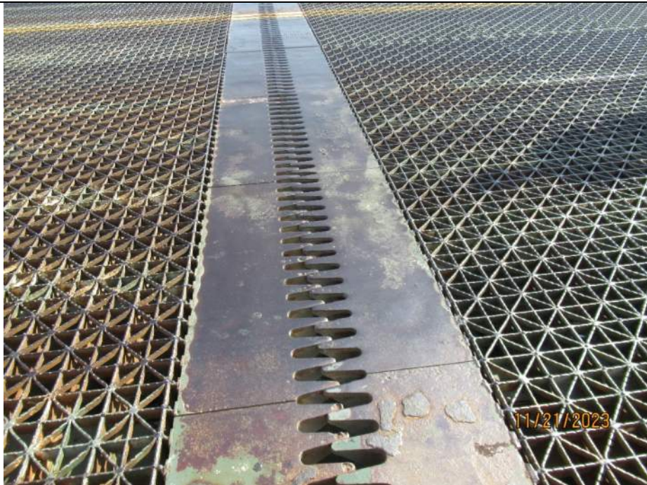
Photo S-138 - [Span 5] -Bascule span center finger joint, general view across SB lanes, Looking East
