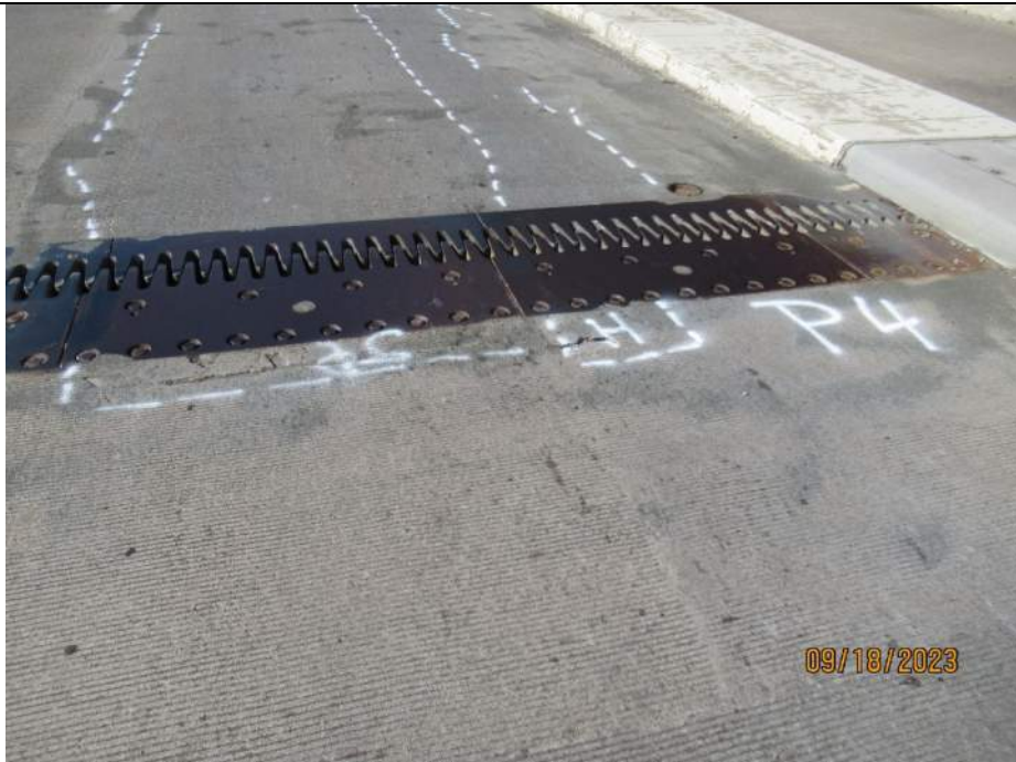
Photo S-48 - [Span 4] -NB right lane detail view of deck cracking, spalling and delamination along finger joint plates, Looking North
