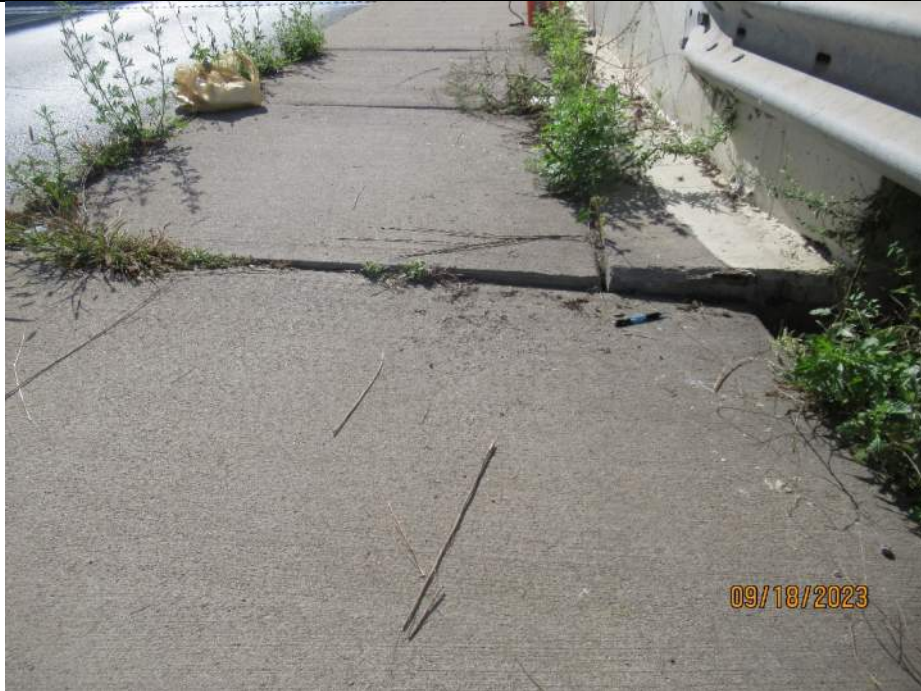
Photo S-25 - [North Approach] -Northwest sidewalk at guard railing transition, settlement on north side at barrier corner up to 3", Looking South
