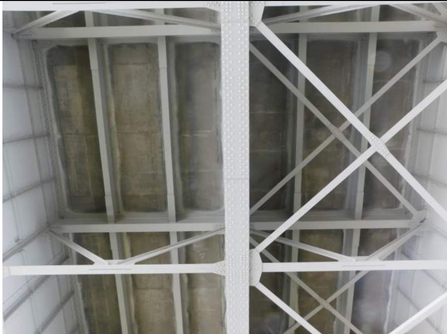
Photo S-158 - [Span 3 ] -Deck underside, general view between Floorbeam 20S-21S, Girders 2W-4W, Looking North
