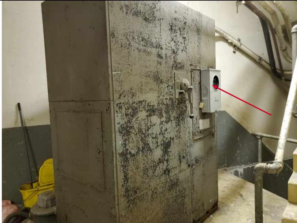
Photo E-01: Abandoned Electrical Equipment on the South Pier. Note the Meter has been removed.
