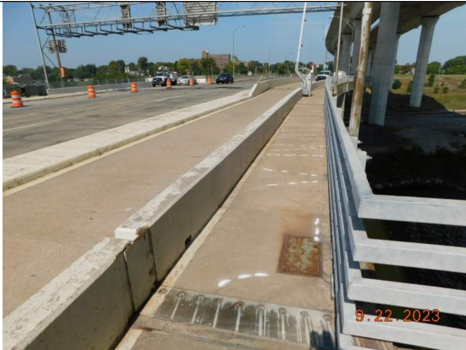
Photo S-114 - [Span 6] -East sidewalk and trail topside, barrier and railings, good condition general view, Looking North
