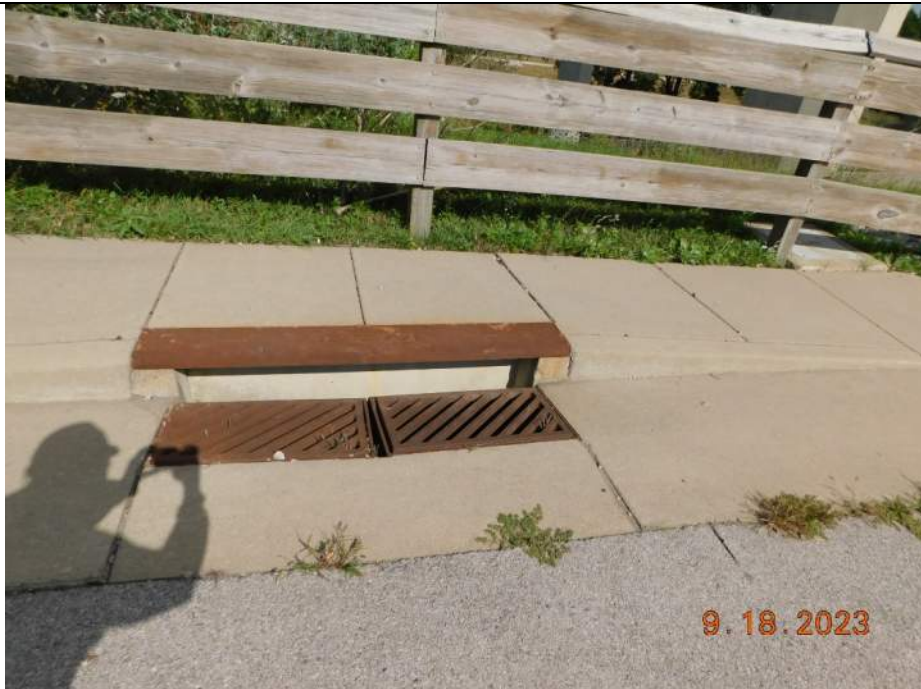
Photo S-34 - [South Approach] -Southeast drain inlet at east side sidewalk / trail is clear, detail view, Looking East
