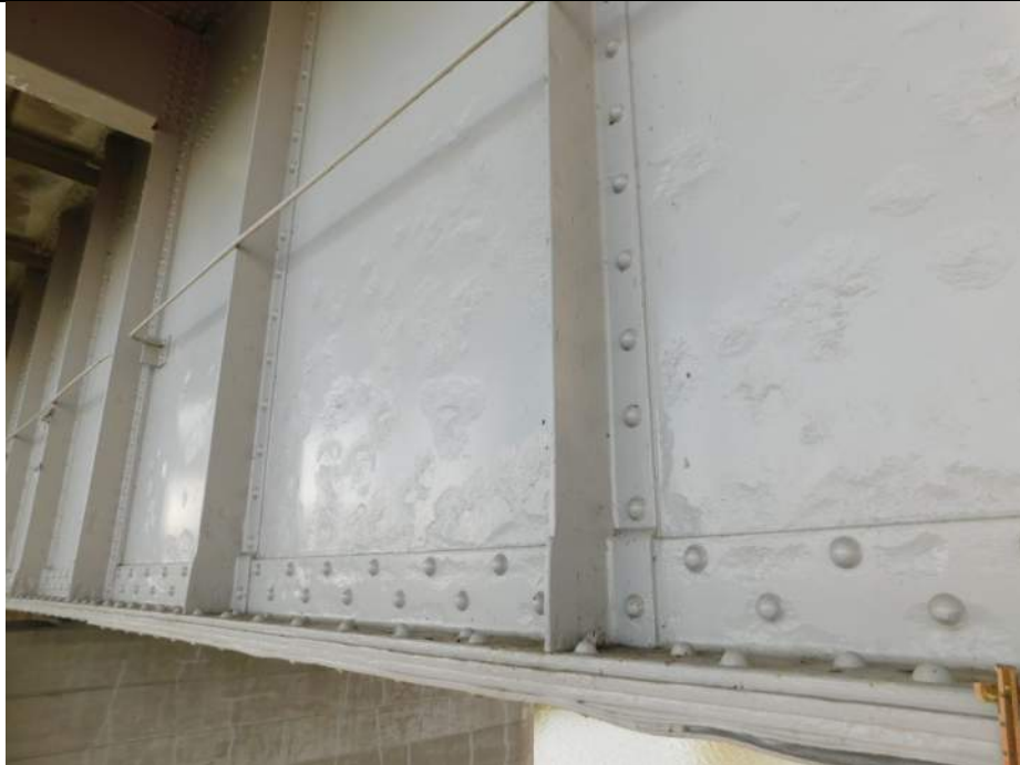
Photo S-175 - [Span 2] -Girder 4W East web, scattered painted over section loss up to 0.125" deep across lower third of web, Looking Southwest
