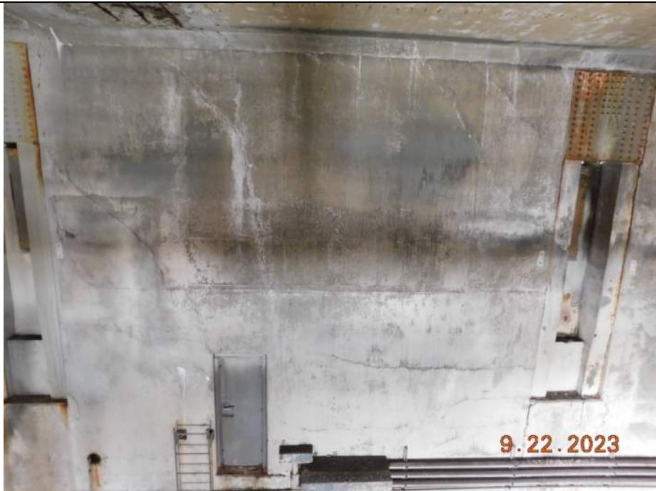
Photo S-344 - [Pier 5 Interior] -Counterweight Pit (Level E), upper North wall diagonal cracking throughout between girder live load bearing cut-outs, Looking North
