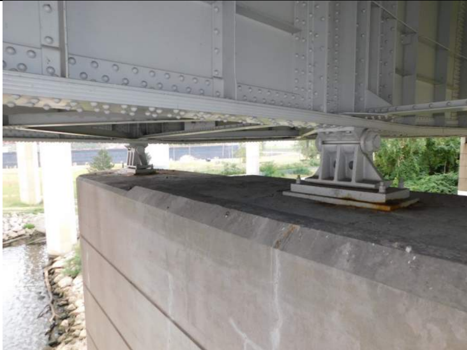
Photo S-255 - [Pier 1] -Bearings 3W and 4W, typical minor tilt to north in contraction, good condition, Looking East
