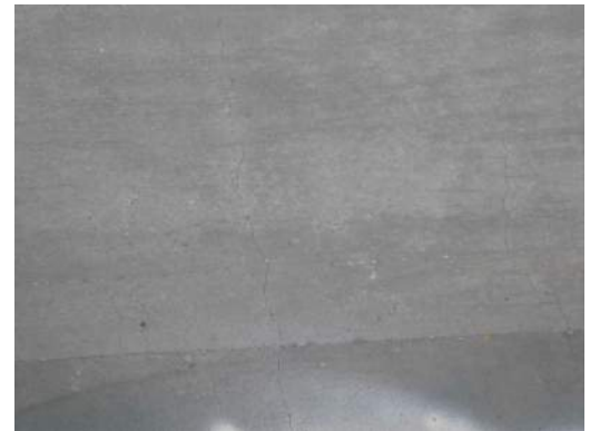
Span 2 deck underside typical shrinkage map cracking
