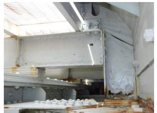
Span 5 sidewalk supports, holes in webs
