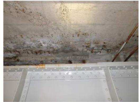
Pier 4 roadway span underside (Level C), deck spalling above G4W
