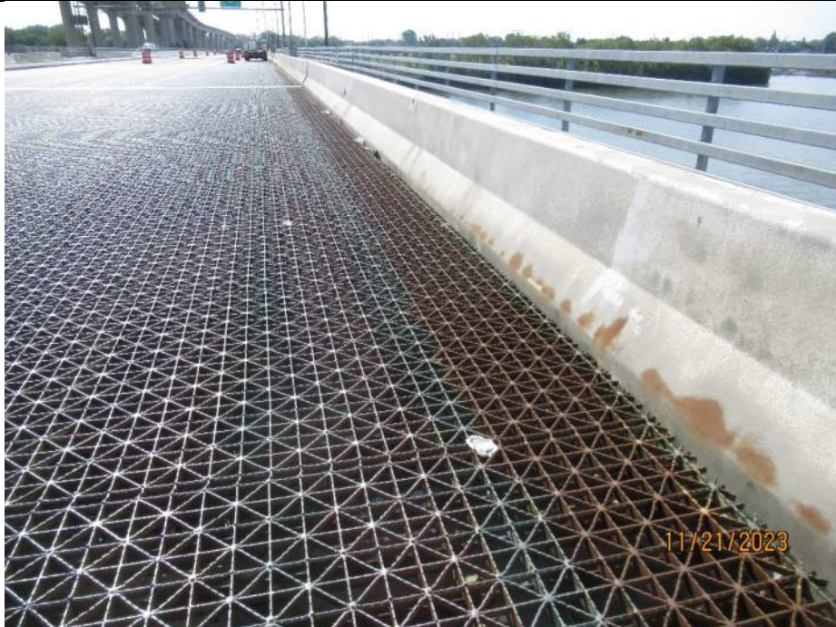
Photo S-91 - [Span 5] -North leaf, West roadway steel barrier, minor corrosion at base, peeling paint throughout, Looking South
