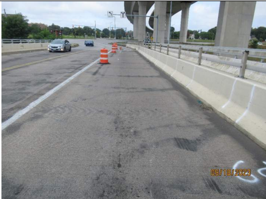
Photo S-66 - [Span 10] -Roadway deck and wearing surface, NB right lane from Pier 9, Looking North
