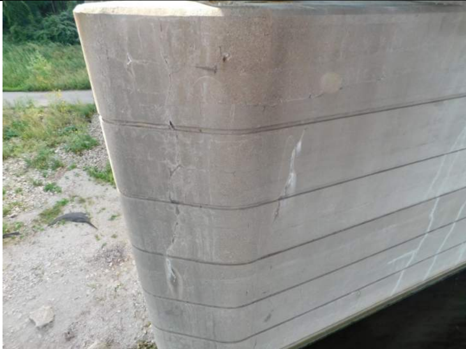
Photo S-287 - [Pier 1] -Pier north side at east end, detail view of vertical cracking, Looking Southwest
