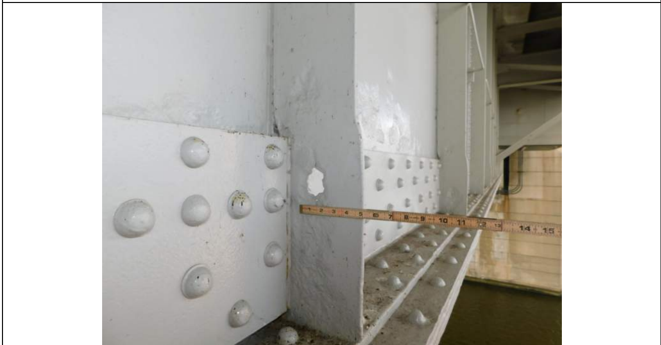
Photo S-182 - [Span 4] -Girder 4W East lower web between FB30S-31S exhibits a 2" diameter hole in the base of the vertical stiffener, Looking Northwest
