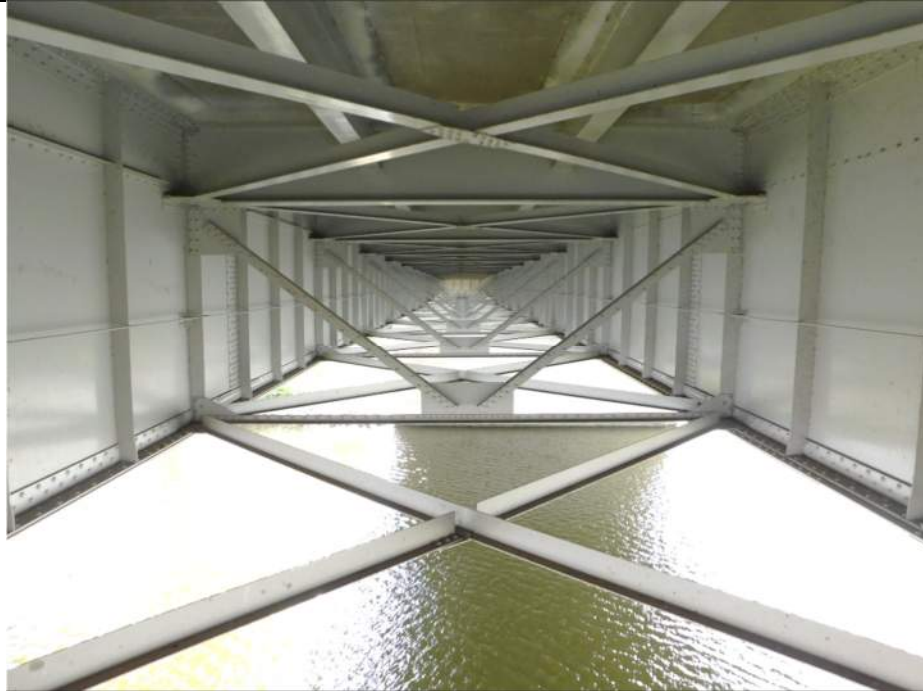
Photo S-207 - [Span 2] -General view of diagonal and transverse bracing between Girders 3W and 4W at Floorbeam 14S, Looking South
