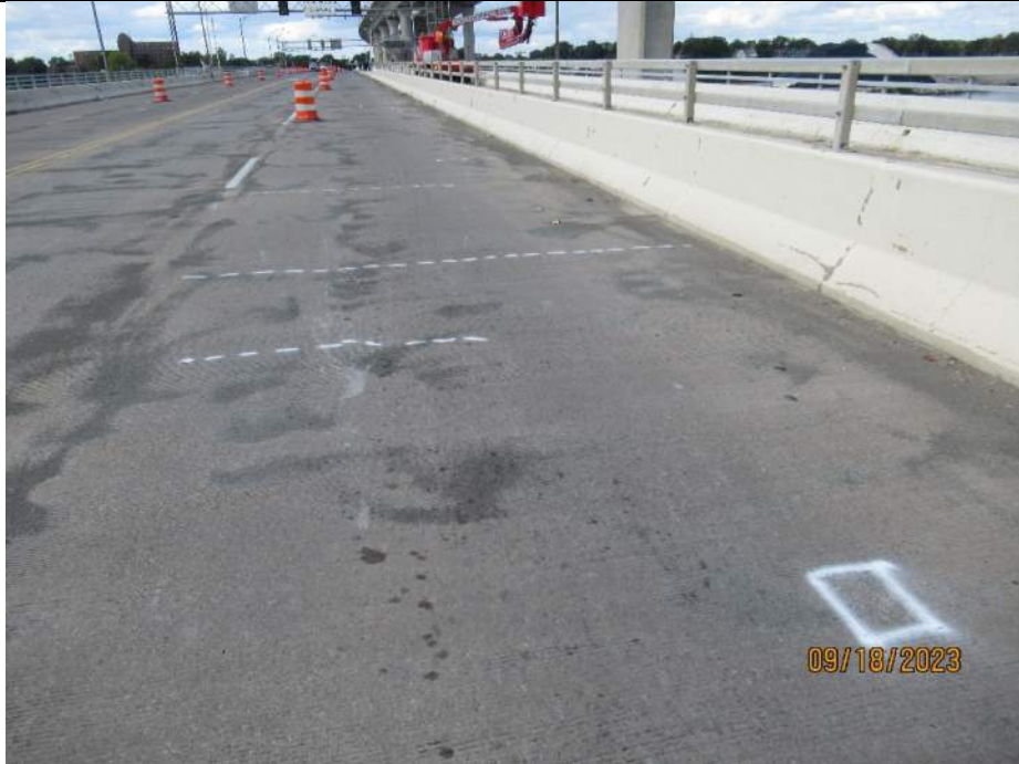
Photo S-43 - [Span 3] -Roadway deck and wearing surface, NB lanes at mid-span, Looking North
