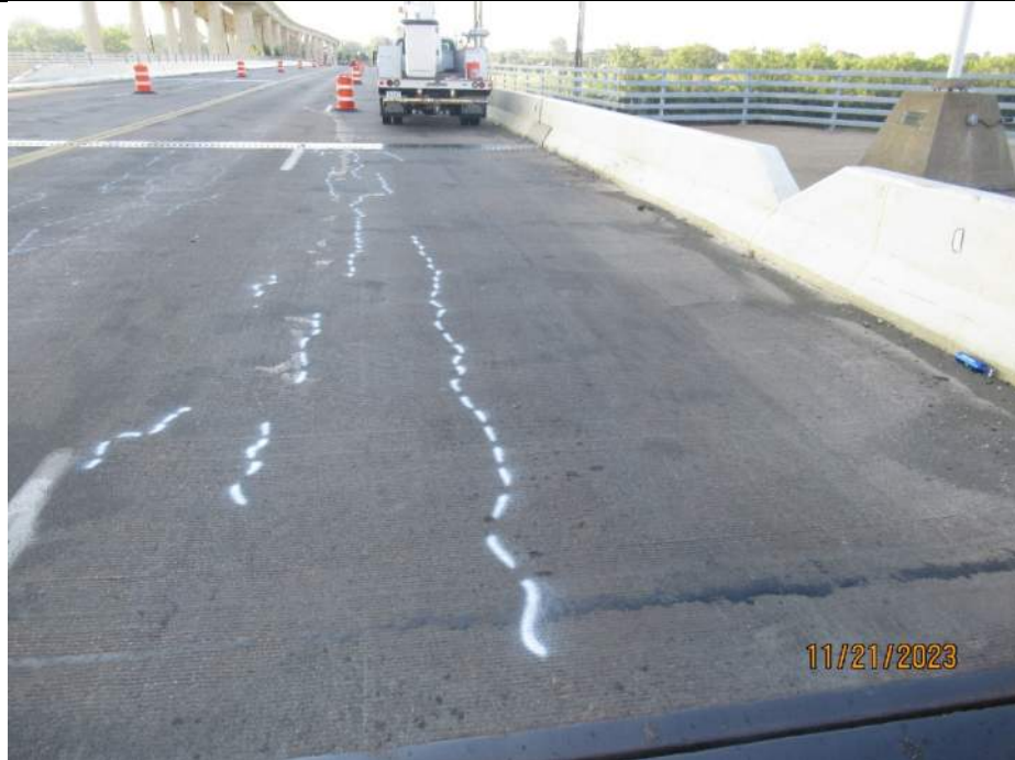
Photo S-51 - [Pier 4 Span] -Roadway deck and wearing surface, SB lanes, Looking South
