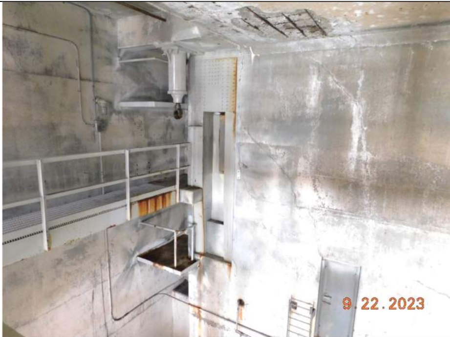
Photo S-348 - [Pier 5 Interior] -Roadway span underside (Level C), view of 4 ft x 3 ft spall to deck underside above counterweight at G1W, Looking Northwest
