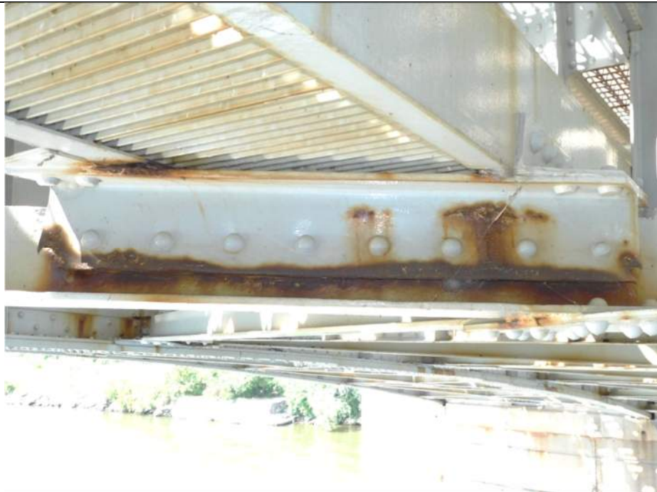
Photo S-252 - [Span 5, North Leaf] -Upper T-section support below center catwalk (G2W-G3W) between FB2n-FB3n at diagonal bracing connection exhibits a pack rust throughout and small edge holes, Looking Northwest
