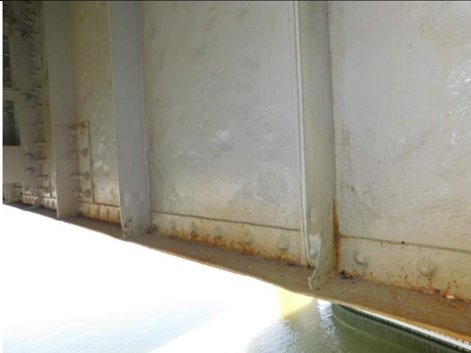
Photo S-225 - [Span 5, South Leaf] -Floorbeam 2s, north face between G3W-G4W, holes in bottom of web stiffeners up to 6" dia. and web reinforcement repair, Looking Northwest
