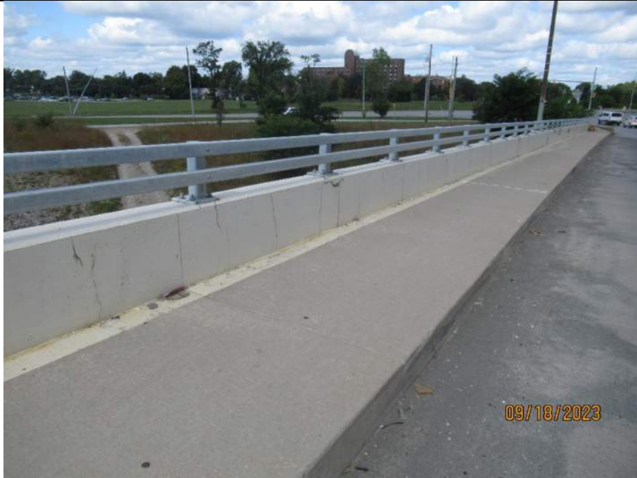
Photo S-119 - [Span 9] -West sidewalk, barrier and railing, minor transverse and vertical cracking, Looking North
