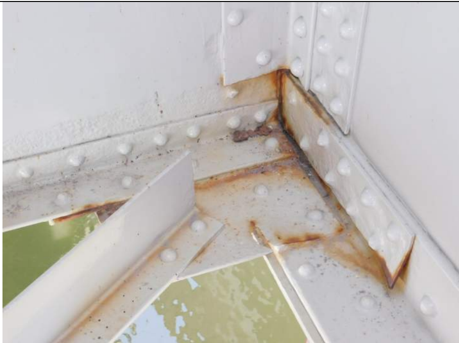
Photo S-244 - [Span 5, North Leaf] -Lower diagonal bracing connection plate with 4" x 1" hole, at south side FB2n and G4W west side connection, Looking North
