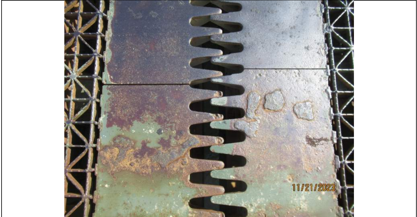
Photo S-139 - [Span 5] -Bascule span center finger joint, detail view of horizontal mis-alignment with fingers in contact, Looking East
