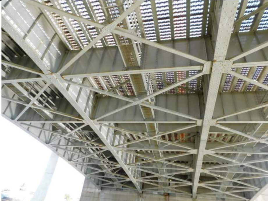
Photo S-165 - [Span 5] -Span framing and underside general view, South leaf, Girders 2W-4W, Looking South
