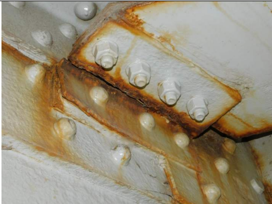
Photo S-240 - [Span 5, South Leaf] -Upper diagonal bracing at FB6s north side to G2W west side, connection angle fully cracked/broken, Looking Southeast
