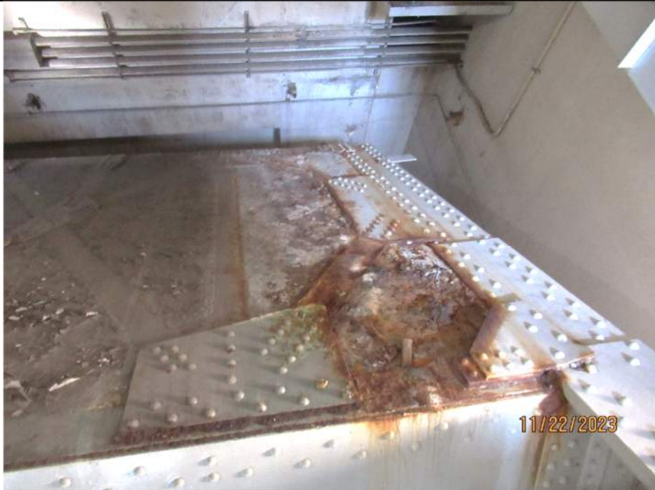
Photo S-362 - [Pier 5 Interior] -Counterweight top at east side (G4W) with moderate corrosion and minor spalling deterioration across the top of the block, Looking North
