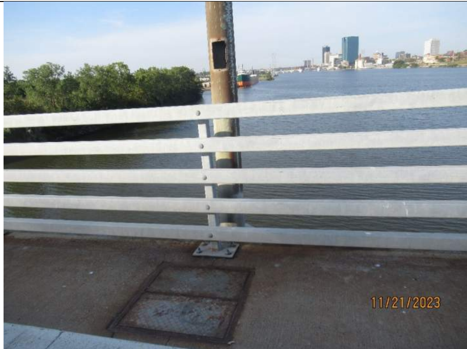
Photo S-317 - [Span 2] -West side light pole, missing access cover above pedestrian railing, typically good condition otherwise, Looking West
