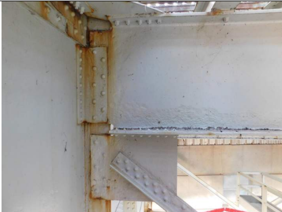
Photo S-218 - [Span 5, South Leaf] -Floorbeam 6s between G1W-G2W, typical section loss to lower web, typical section loss to K-bracing connection plate below, Looking South
