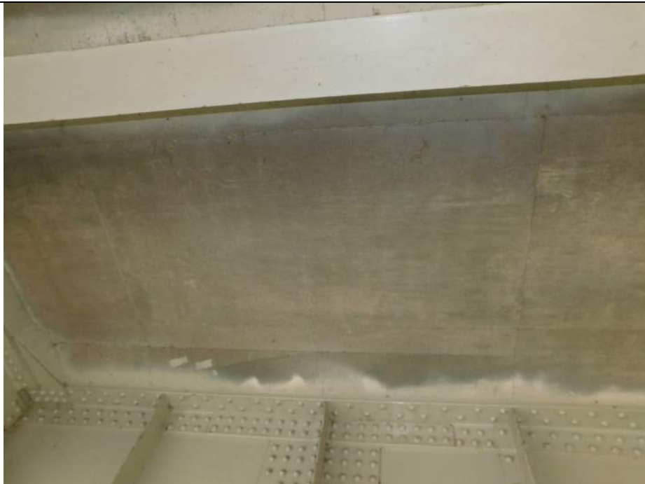
Photo S-154 - [Span 2] -Deck underside, detail view between Floorbeams 6S & 7S, Girder 2W and Stringer 3W, Looking West
