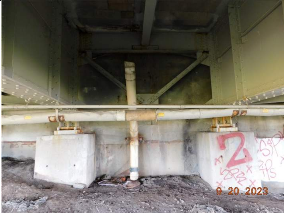
Photo S-269 - [North Abutment] -Bearings 2W and 3W, typical minor rust stains and bleeding corrosion to rockers and masonry plates, Looking North
