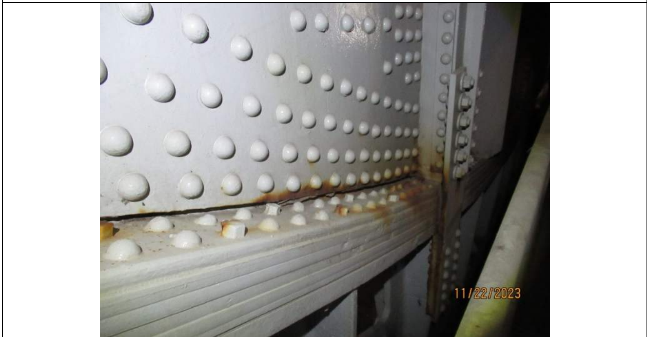
Photo S-358 - [Pier 5 Interior] -Girder 3W, West face behind the trunnion bearing, typical localized minor corrosion to plate edge above bottom flange, Looking East
