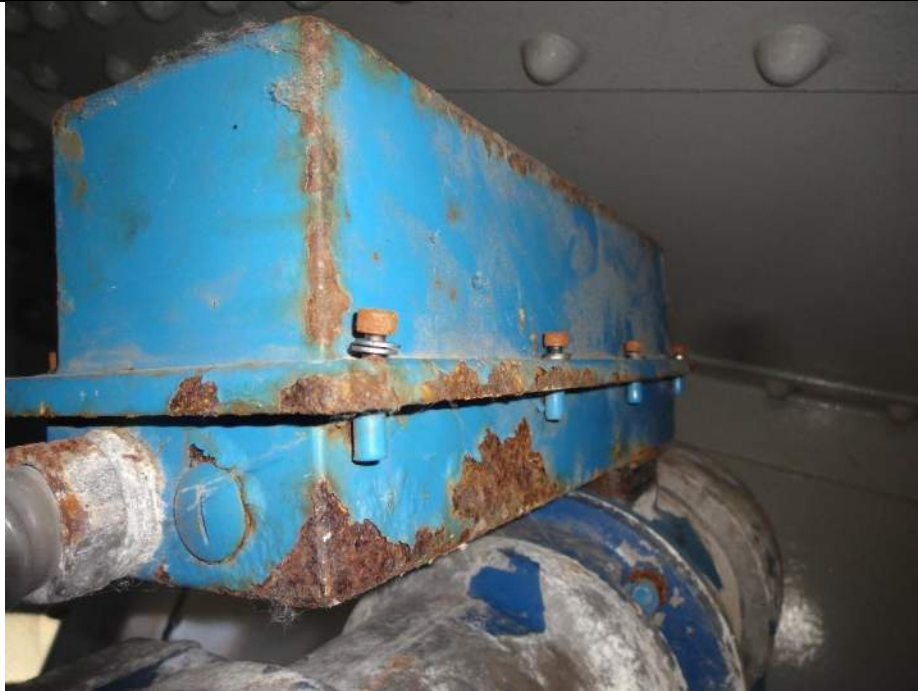
Photo 73 - [SE Swing Gate] – Note loose fasteners on RACO limit switch housing for swing gate.
