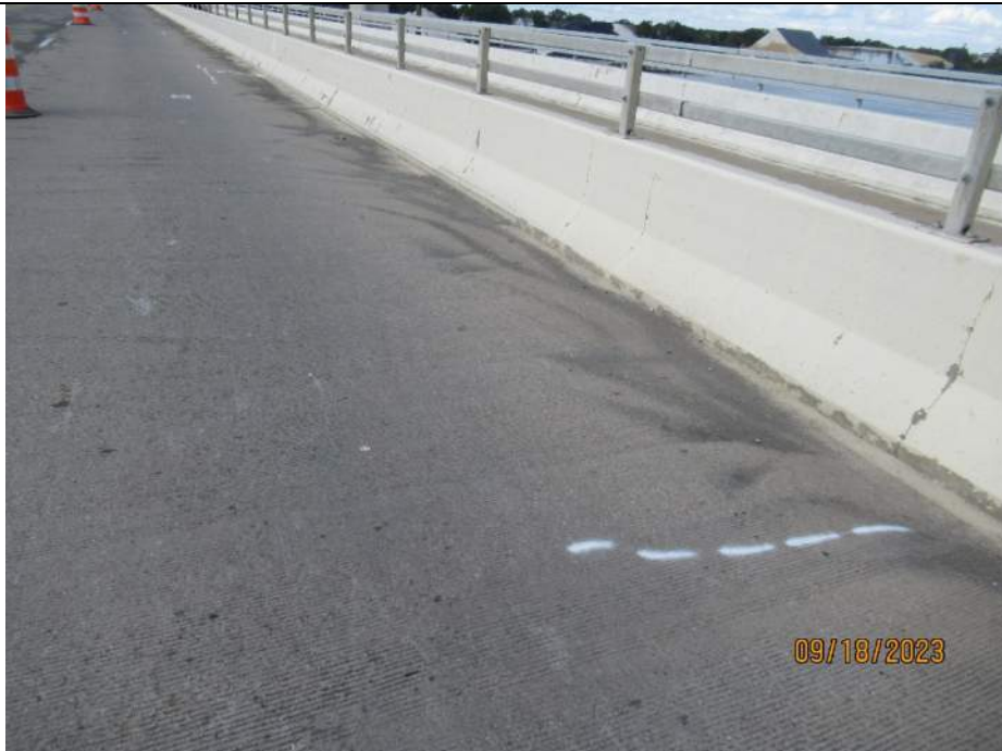
Photo S-84 - [Span 2] -East roadway barrier, typical full height vertical cracking, Looking East
