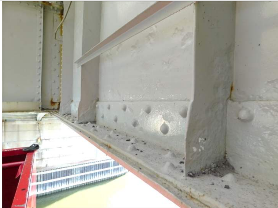
Photo S-210 - [Span 5, South Leaf] -Girder 2W, east side between FB1s-FB2s, typical section loss and small holes in base of stiffener, Looking Southwest
