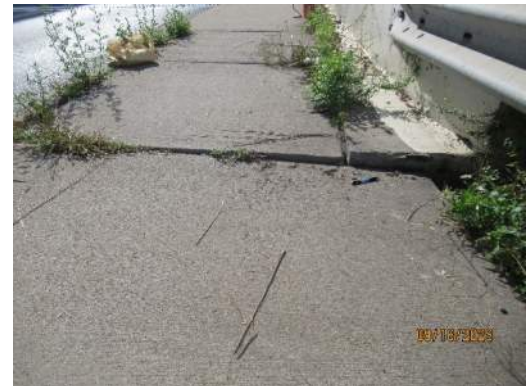
Northwest sidewalk settlement at transition
