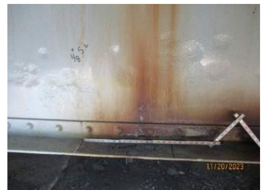
Span 8 FB20s south BF and web SL
