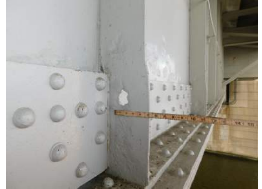
Span 4 Girder 4W stiffener hole
