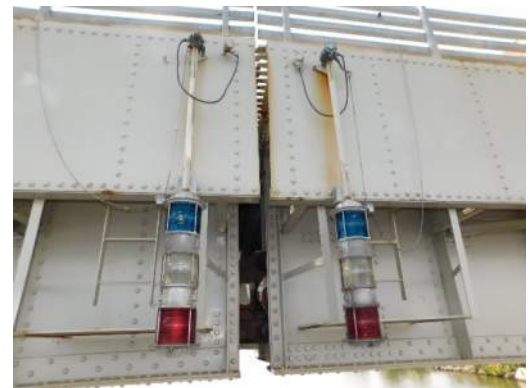
Span 5 East side navigation lights
