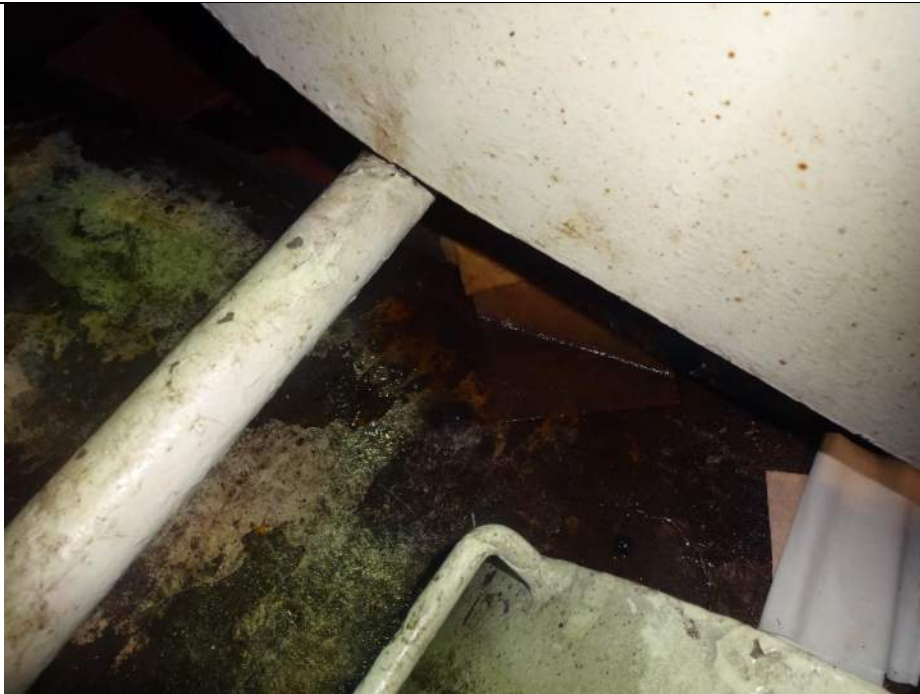
Photo 6 - [North Machinery Room] – Note oil leak from chain housing.
