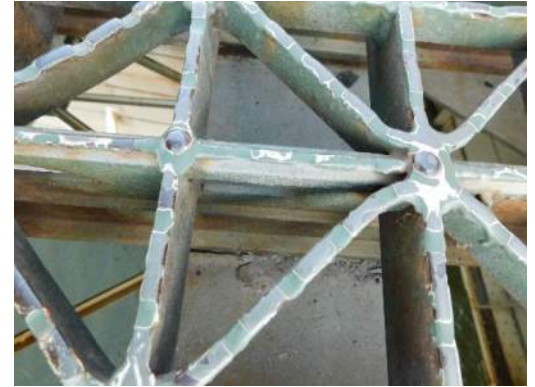
Grid deck main bar to stringer top flange broken welds
