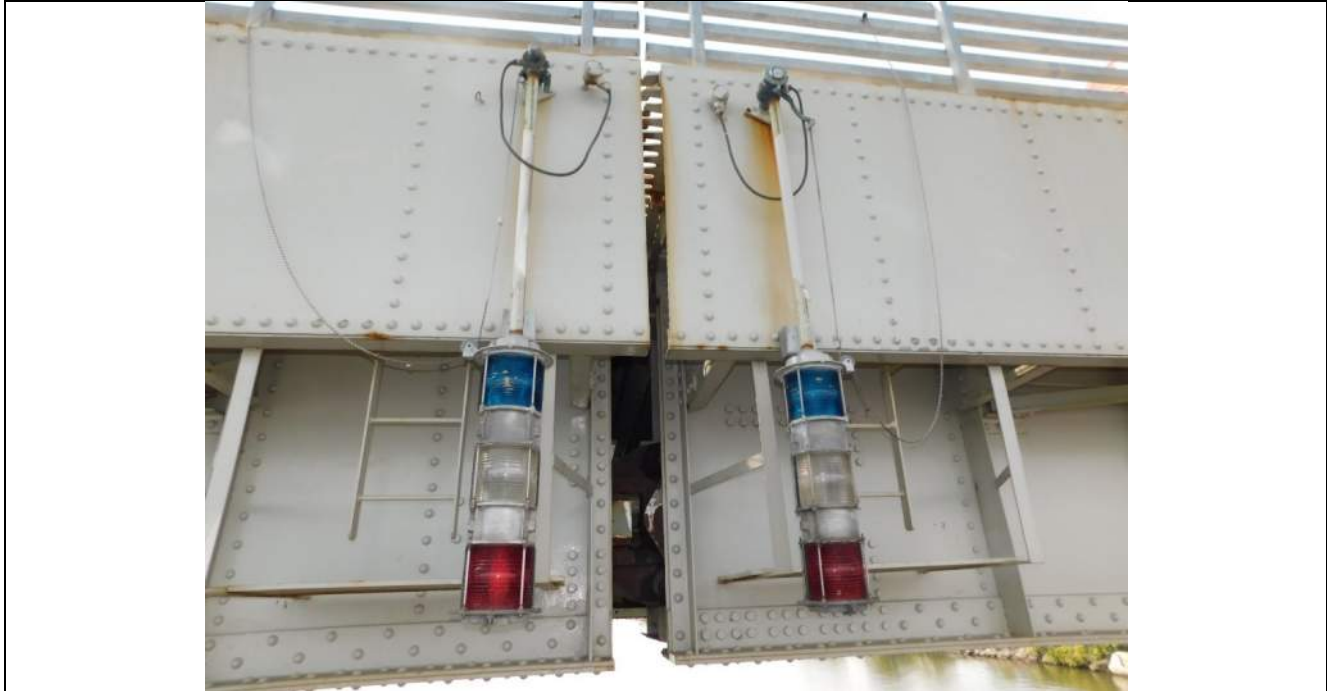
Photo S-321 - [Span 5] -East side navigational lights, good condition, lights not functional, Looking West
