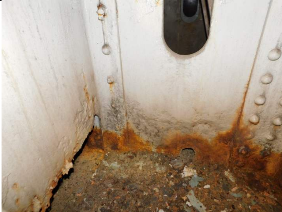
Photo S-351 - [Pier 4 Interior] -Trunnion Tower 3W West leg interior at base, active section loss and corrosion hole in diaphragm, Looking Northeast
