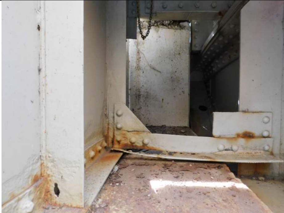
Photo S-247 - [Span 5, South Leaf] -East sidewalk support and fascia girder, typical section loss and corrosion hole in support angle and stiffener across from FB7s, Looking South
