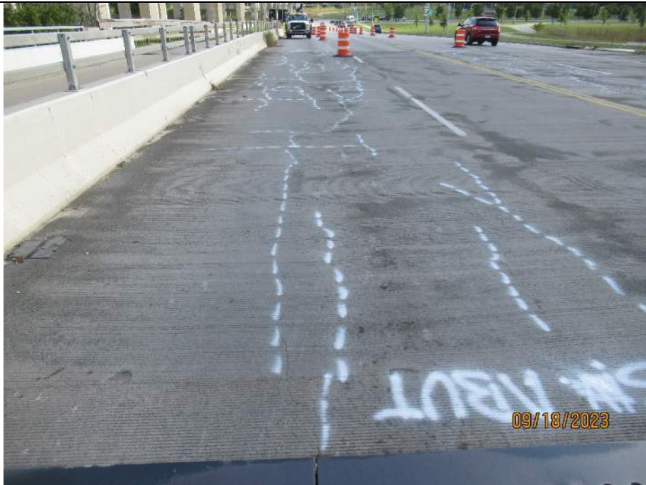
Photo S-10 - [South Approach] -Roadway approach slab, NB right and left general view, Looking South
