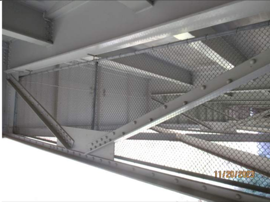
Photo S-339 - [Span 10] -Security fencing along Floorbeam 6S is in good condition, including connections to floorbeams, girders, bracing members, view between G1W-G2W, Looking Northwest
