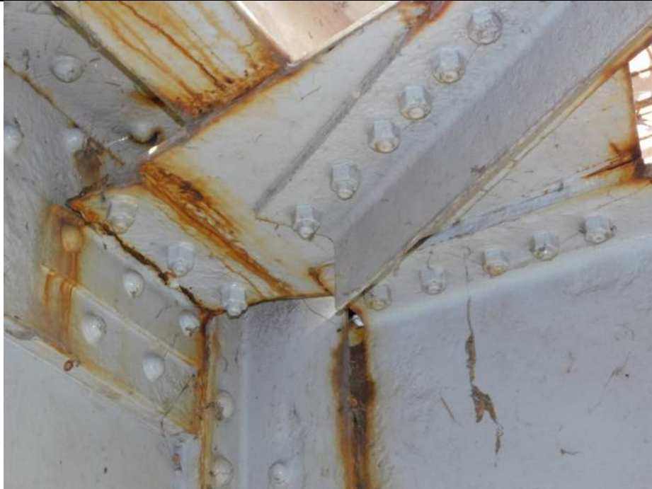
Photo S-239 - [Span 5, South Leaf] -Upper diagonal bracing at FB6s south side to G3W west side, connection angle fully cracked/broken, Looking Northwest
