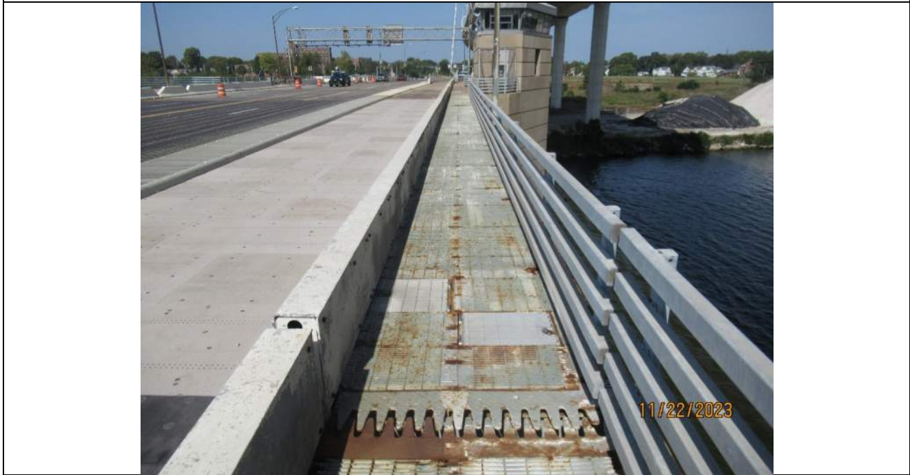
Photo S-110 - [Span 5] -North leaf east sidewalk and railing, typical good condition of rail and widespread minor corrosion to sidewalk grating, Looking North
