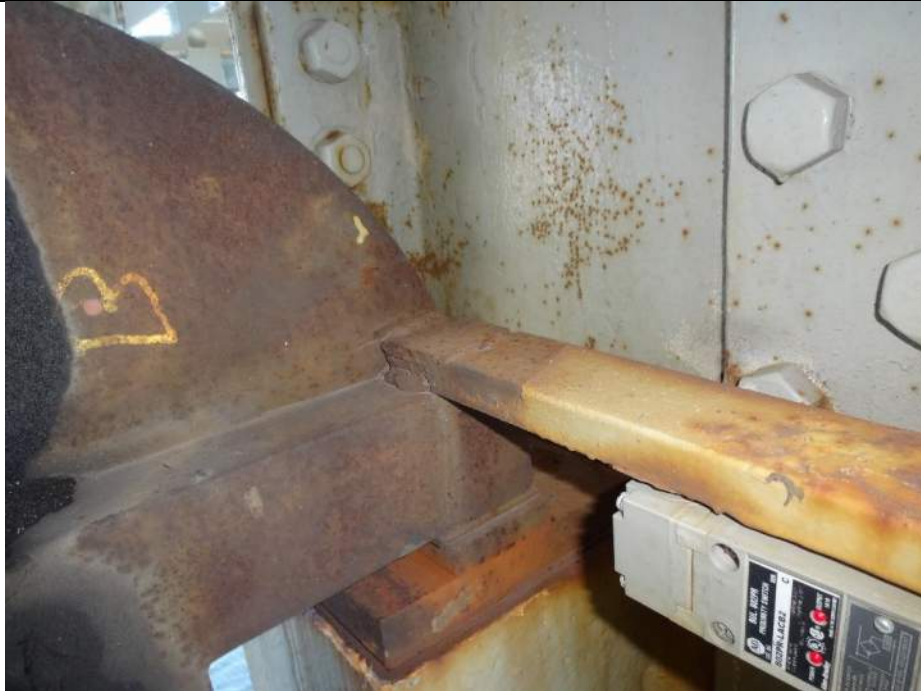
Photo 51 - [NE Outboard Locking Mechanism] - Limit switch targets have poor welds on locking mechanism.
