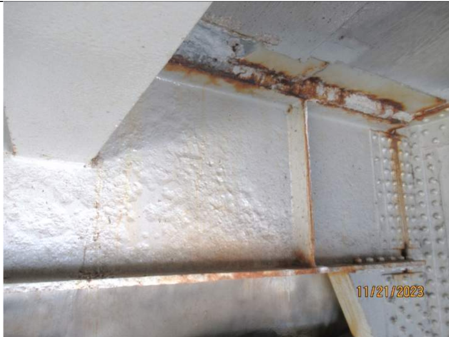
Photo S-187 - [Span 1] -Floorbeam 0S at the South Abutment widespread painted over deep section loss to the web and flanges, area next to Girder 2W, Looking South
