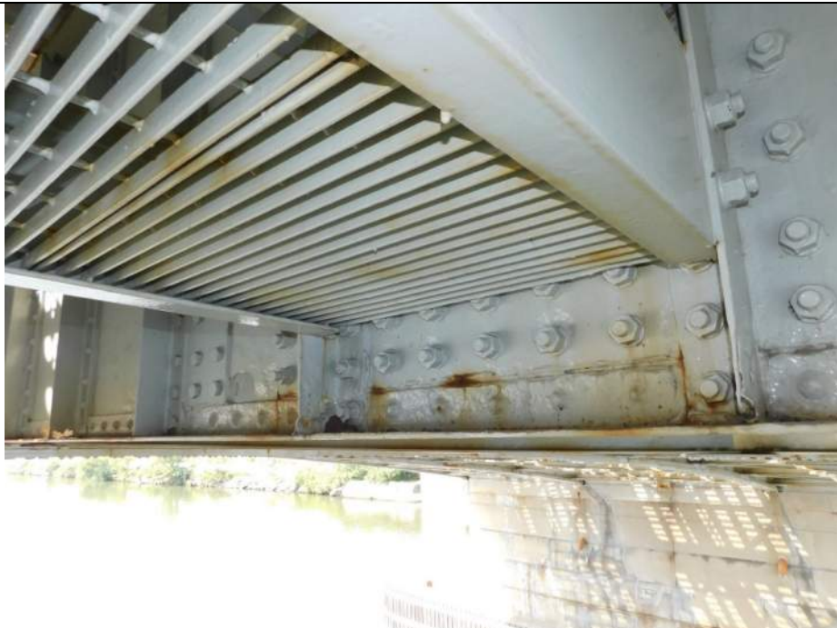
Photo S-224 - [Span 5, South Leaf] -Floorbeam 2n, south face between G3W-G4W, holes in bottom of web stiffeners up to 4" x 1", Looking Northwest
