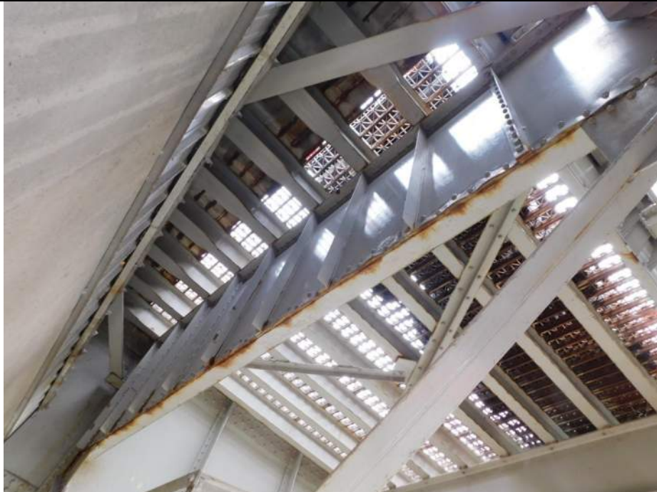
Photo S-232 - [Span 5, North Leaf] -Floorbeam 7n between G1W-G2W, packing corrosion with warping to bottom of web plate along north face, Looking East
