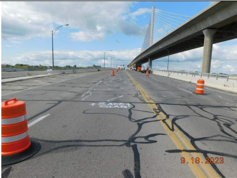
Photo S-6 - [South Approach] -View onto structure from South Approach, Looking North
