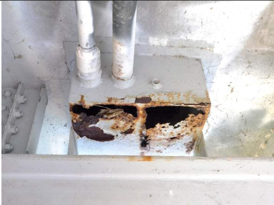
Photo S-332 - [Span 3] -Electrical junction box above Floorbeam 18S East exterior, holes in box, Looking South
