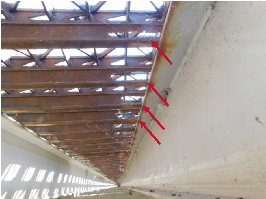
Photo S-57 - [Span 5] -Detail view of grid deck with corrosion holes in lower main bars above Stringer 17W between FB5n-6n, Looking South
