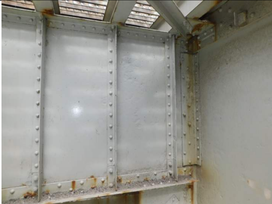
Photo S-233 - [Span 5, North Leaf] -Floorbeam 7n between G1W-2W, typical web and bottom flange section loss, debris at bottom flange, repairs to bases of web stiffeners, Looking South
