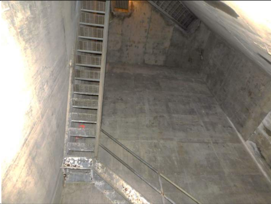
Photo S-370 - [Pier 4 Interior] -Basement Level, Room 1W, access staircase with moderate degradation of galvanizing and minor spot corrosion, Looking South
