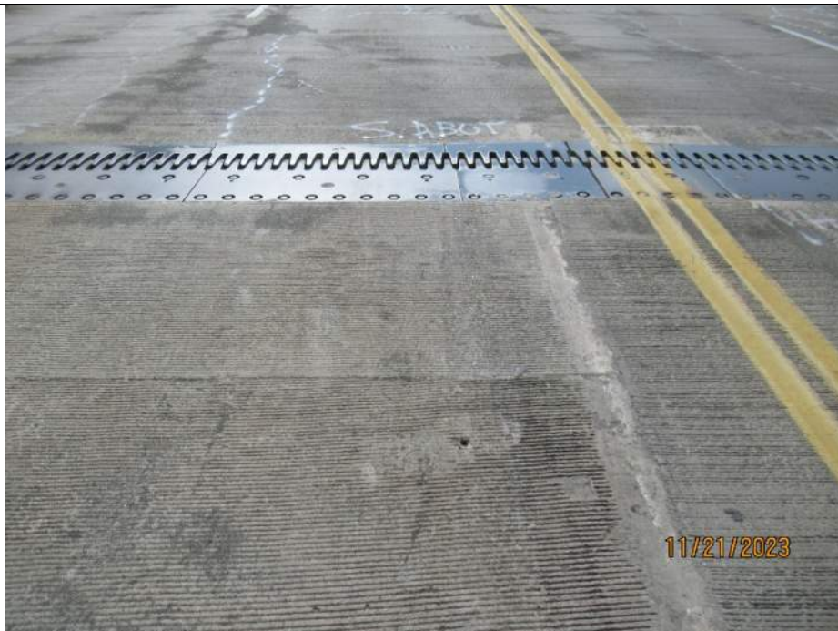
Photo S-126 - [South Abutment] -Abutment reference line finger joint at middle lanes, view showing approach (south) fingers up to 0.75" higher than span (north) fingers, Looking South
