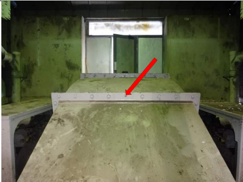
Photo 20 - [North Machinery Room] – Fastener is missing on the seam of central gear enclosure.
