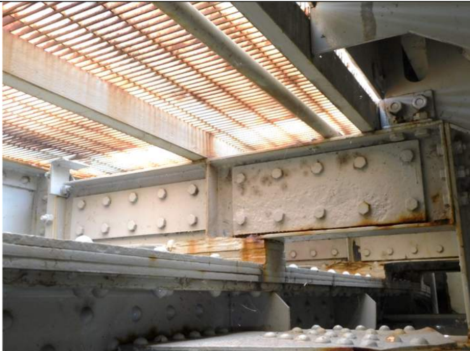
Photo S-248 - [Span 5, South Leaf] -East sidewalk support beams with reinforcement repairs over corrosion holes in webs at FB7s, Looking South
