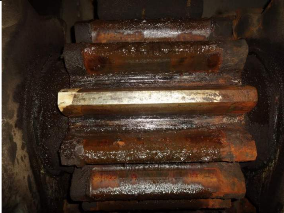
Photo 27 - [SE Corner of South Machinery Room] - Moderate surface corrosion exists on opening and closing faces of teeth as well as rust build up near the edges.
