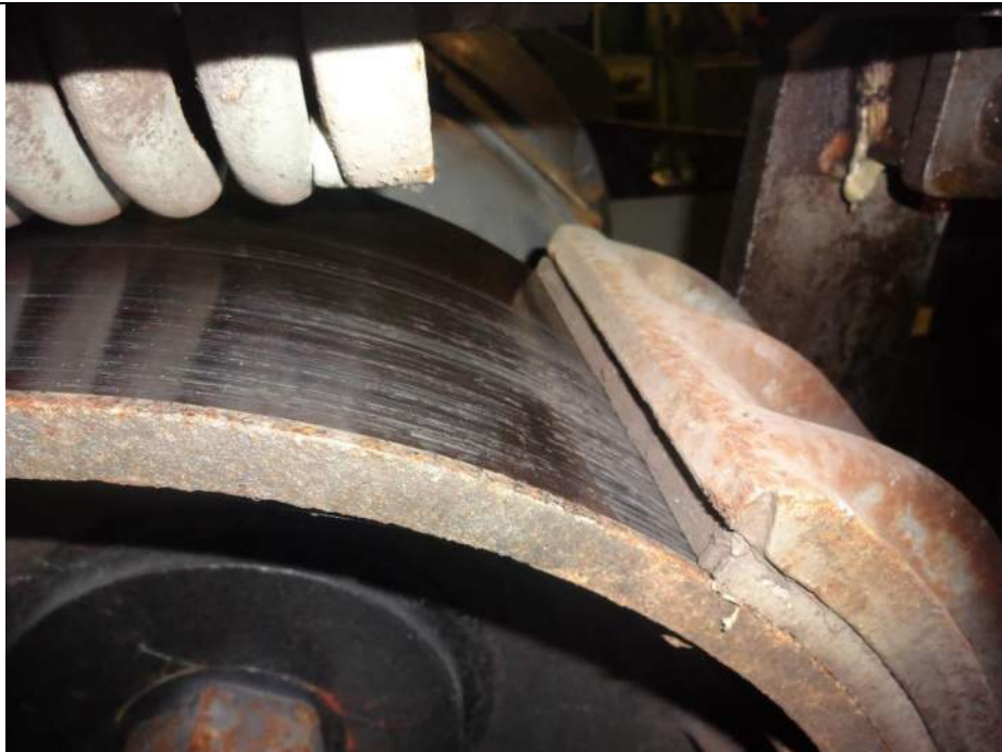
Photo 8 - [North Machinery Room] - Scoring and rust contamination is on brake wheel surface.
