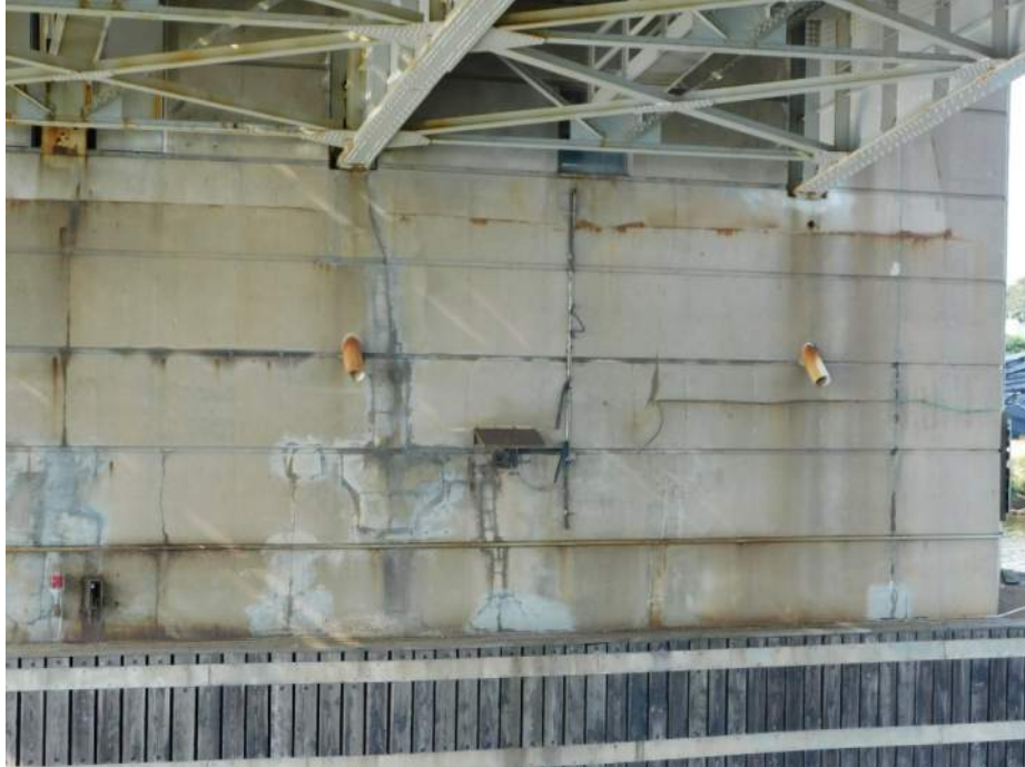
Photo S-303 - [Pier 5] -Detail view of repairs and cracking across east half of south face, Looking North
