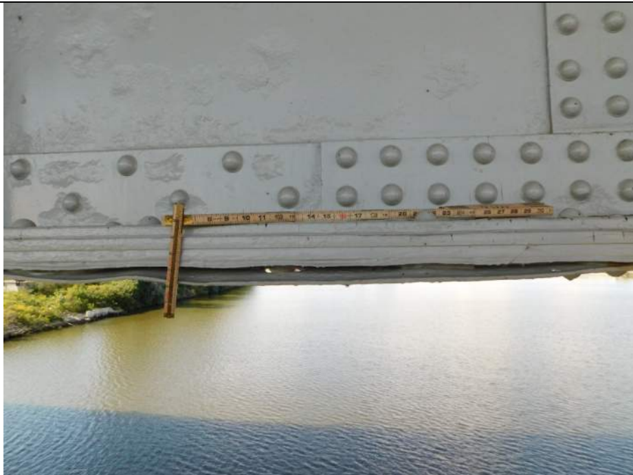
Photo S-176 - [Span 2] -Girder 4W East bottom flange, cleaned packing corrosion with section loss to the plate, Looking West
