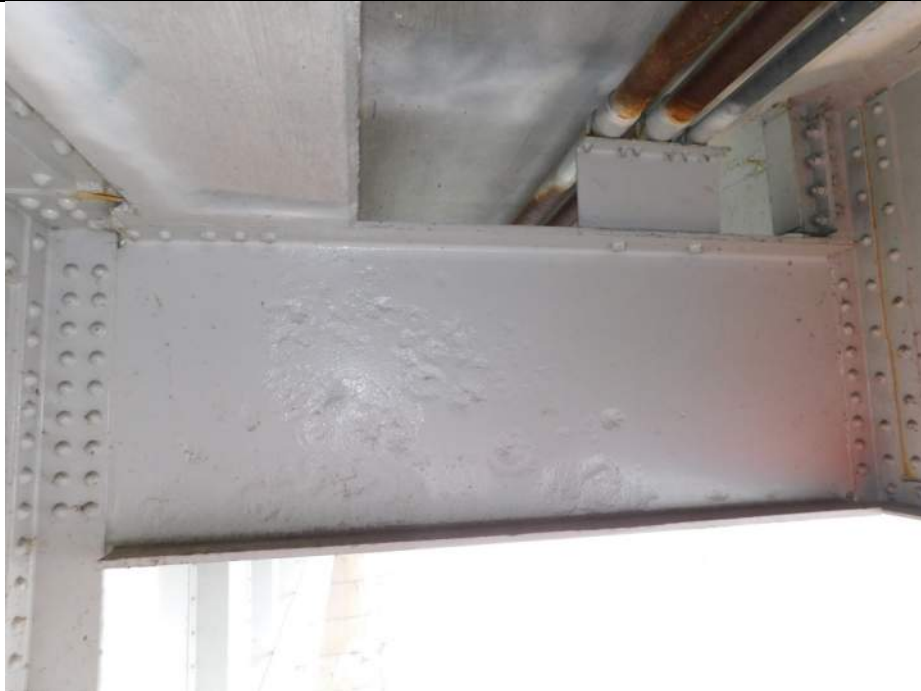
Photo S-199 - [Span 3] -Floorbeam 20S, West exterior, North face, typical painted over section loss up to 0.125" deep across lower web, additional similar loss in middle web, Looking South
