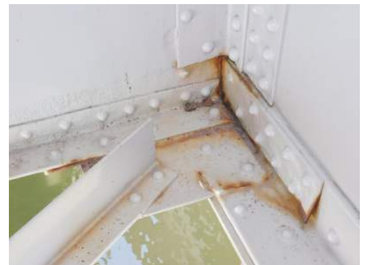
Span 5 lower diagonal connection plate hole
