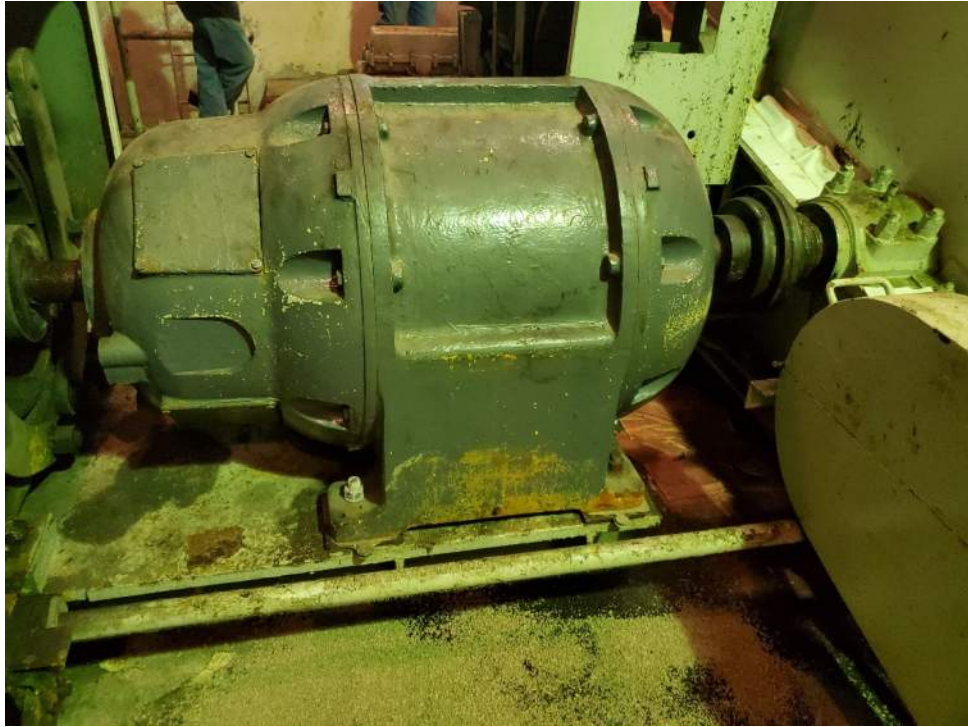
Photo E-09: Southeast Main Drive Motor
