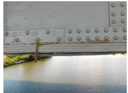
Span 2 Girder 4W east BF pack rust & SL
