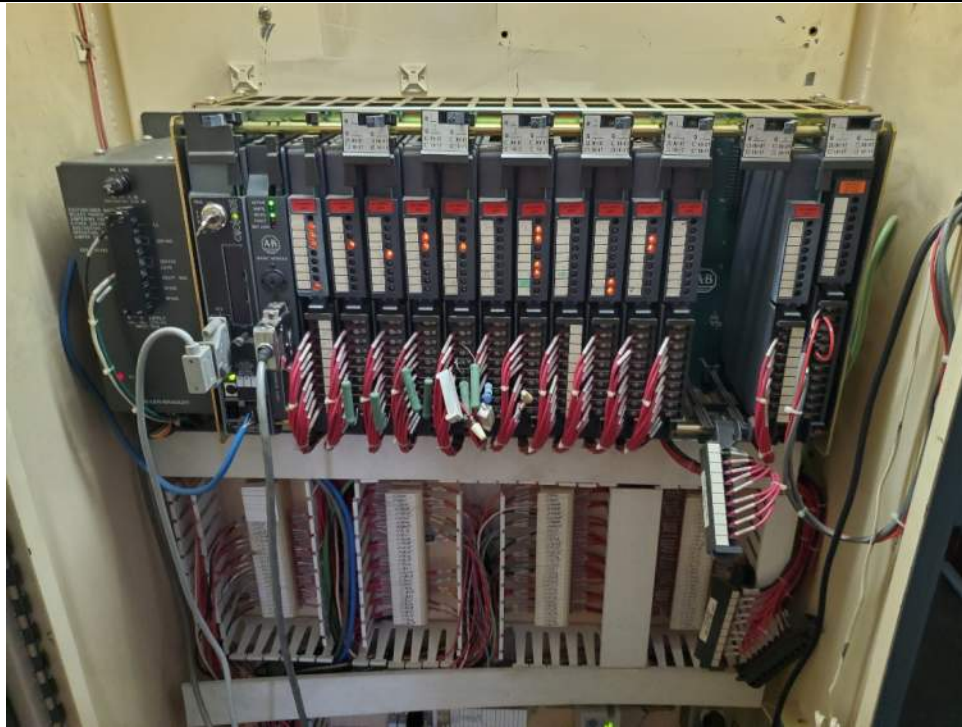
Photo E-15: PLC
