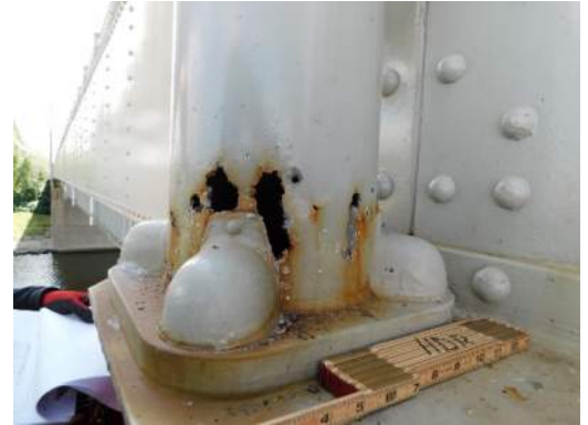
Span 3, FB18s East side light pole base with holes
