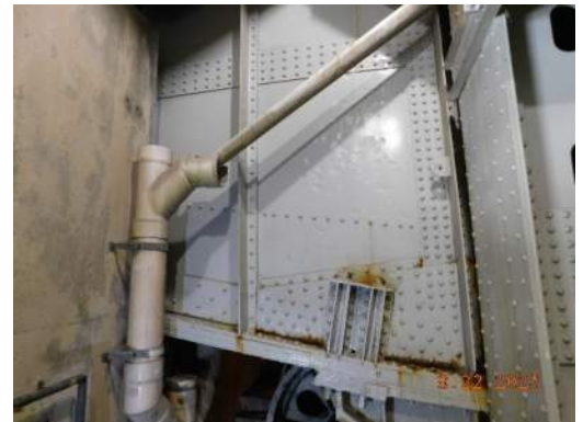
Pier 5, G3W East face widespread painted over section loss
