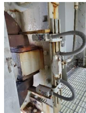
Photo E20: Span Lock Proximity Switch
