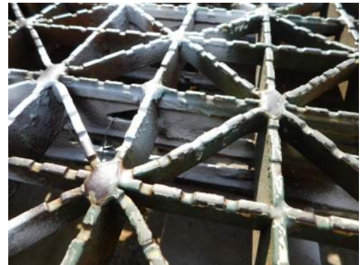
Grid deck main bar corrosion holes
