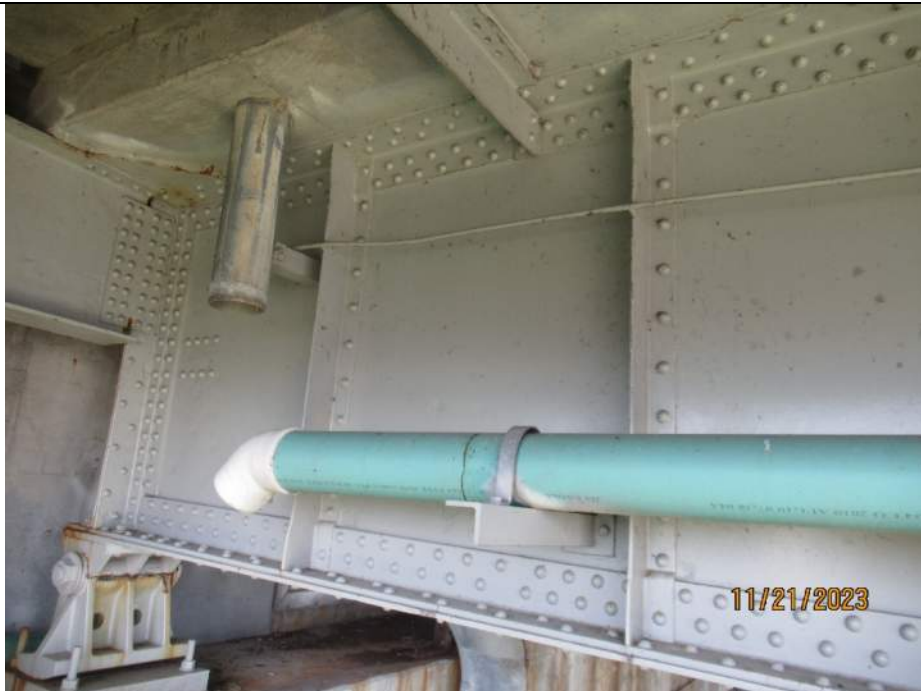
Photo S-150 - [Span 1] -Downspouts at South abutment and east side of span are disconnected at the abutment, Looking Southwest
