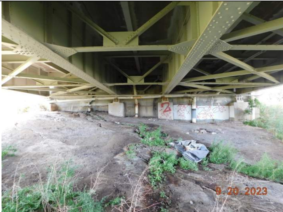
Photo S-278 - [North Abutment] -Abutment columns and back wall general view, Looking North
