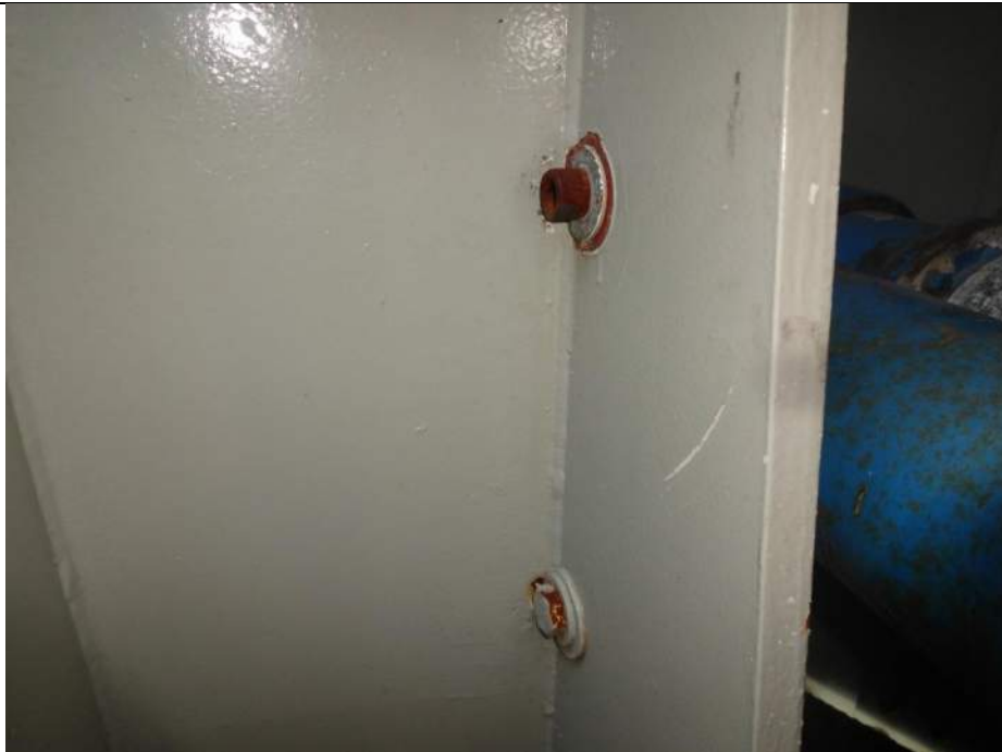
Photo 78 - [NW Swing Gate] - Mismatched actuator bolts are being used on swing gate.
