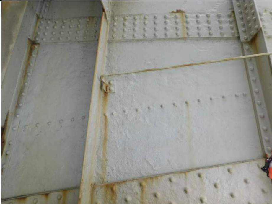
Photo S-213 - [Span 5, North Leaf] -Girder 2W, west face below FB7n, typical widespread section loss to web, splice plates, rivets, stiffeners and bottom flange angle, Looking East
