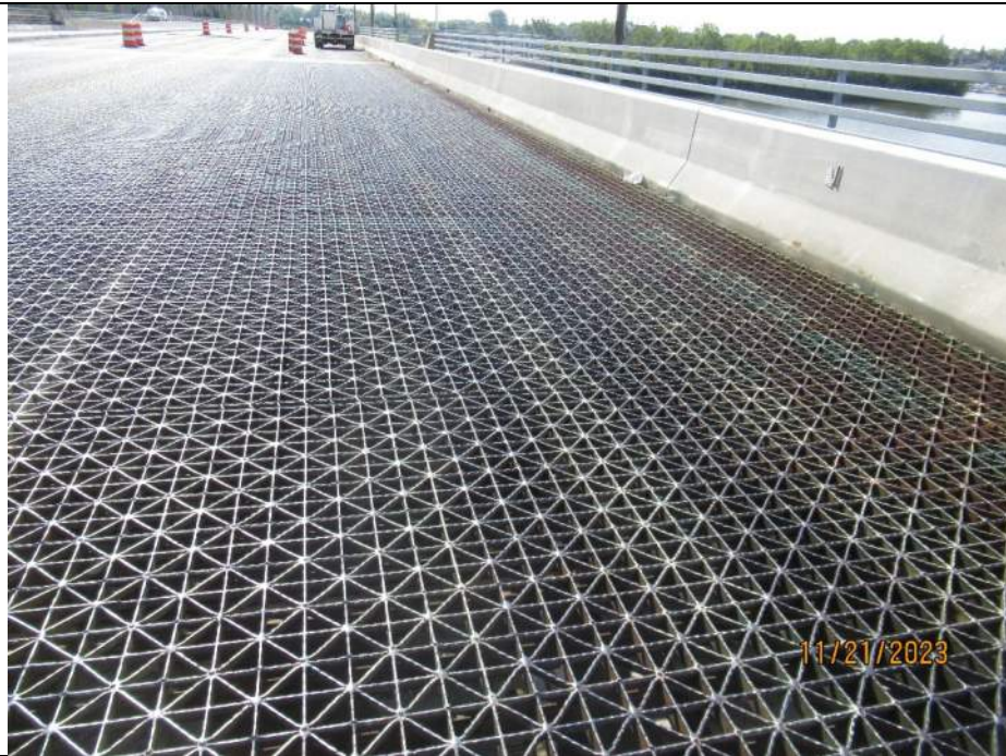
Photo S-52 - [Span 5] -South leaf SB lanes general view of grid deck and roadway barrier, Looking South
