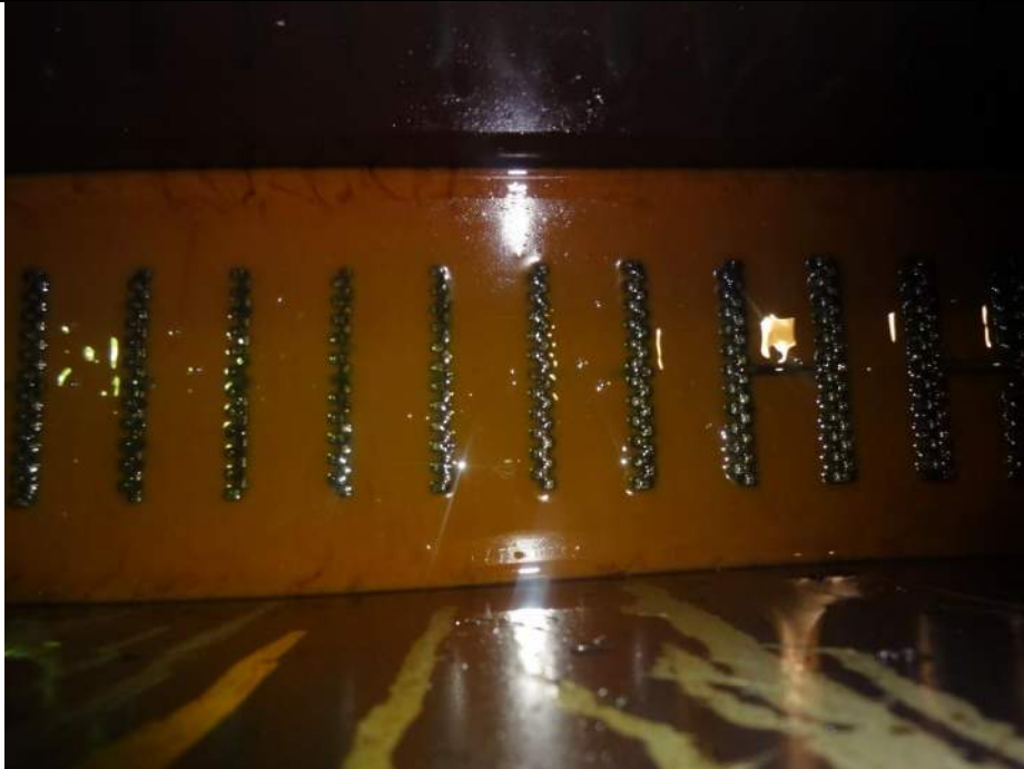
Photo 5 - [North Machinery Room] - Oil in chain housing is contaminated with dirt and debris.
