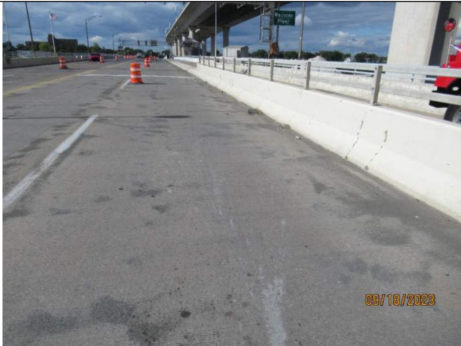
Photo S-46 - [Span 4] -Roadway deck and wearing surface, NB lanes south of mid-span, Looking North
