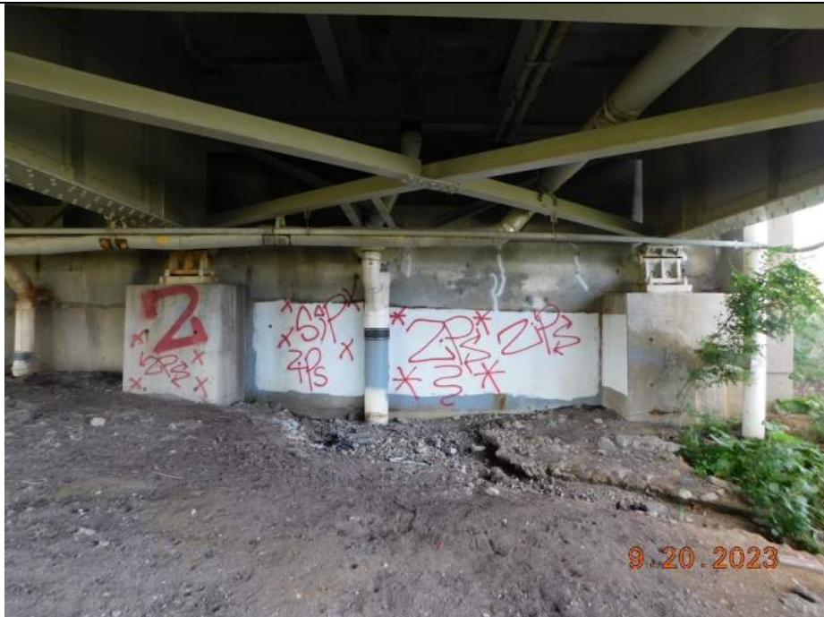
Photo S-280 - [North Abutment] -Abutment columns and back wall view between Girders 3W and 4W, Looking North
