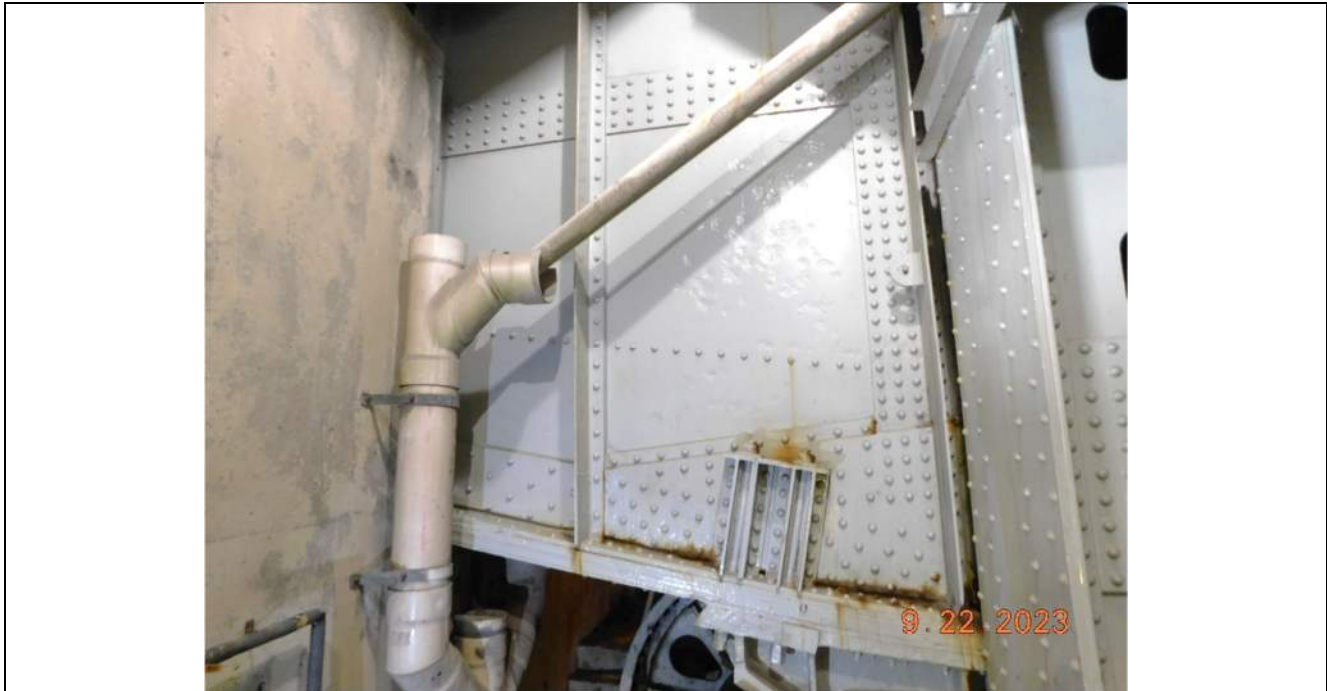
Photo S-359 - [Pier 5 Interior] -Girder 3W, East face between pier wall and trunnion tower, typical painted over section loss to web plate and minor corrosion along bottom flange, Looking West
