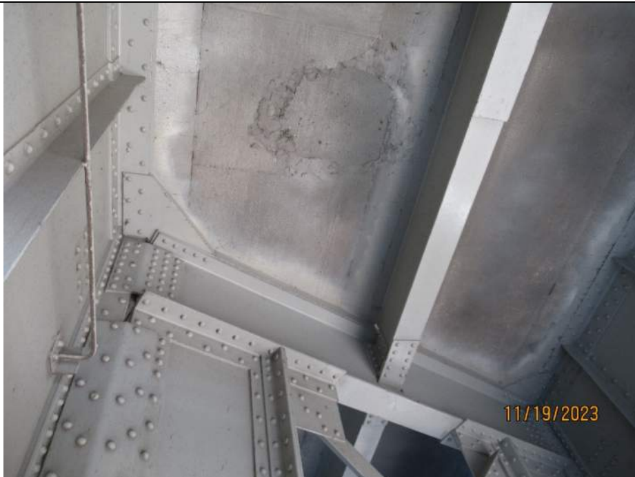
Photo S-160 - [Span 7] -Deck underside, between Girders 2W-3W south of FB14S, isolated patch repair in deck, Looking North
