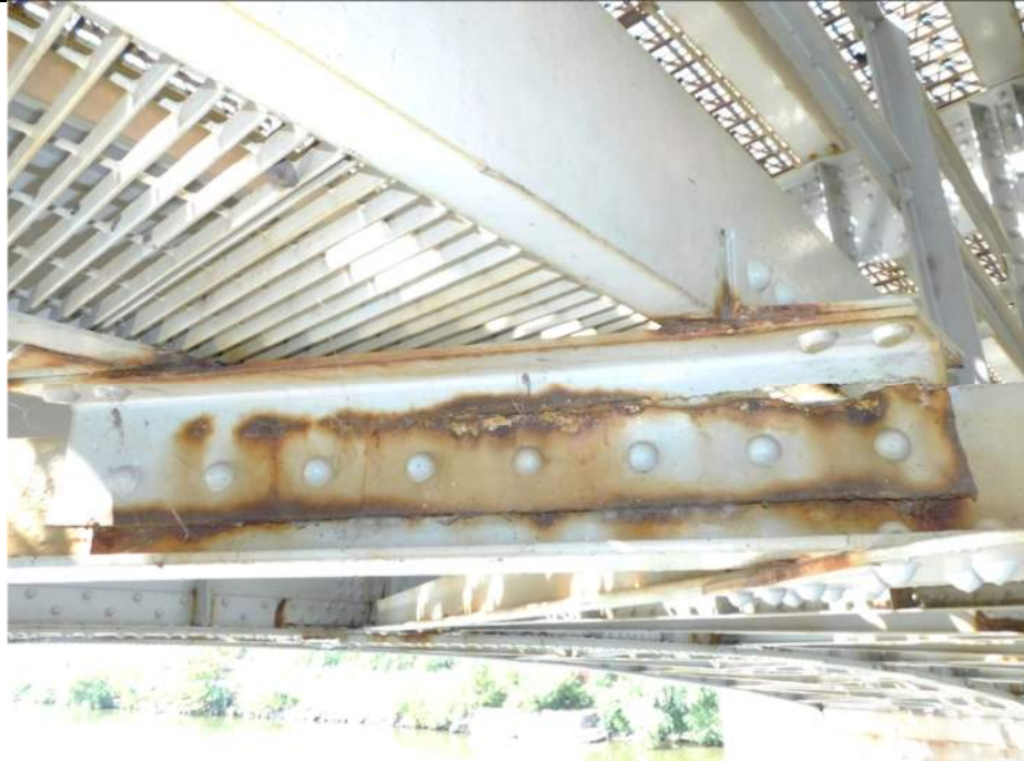
Photo S-251 - [Span 5, North Leaf] -Upper T-section support below center catwalk (G2W-G3W) between FB1n-FB2n at diagonal bracing connection exhibits a 31" L x 1" H corrosion hole in the web with pack rust throughout, Looking Northwest
