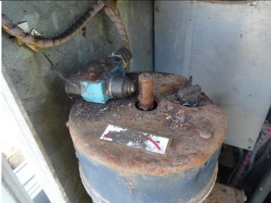
Photo 65 - [NE Traffic Gate] – Note the heavy corrosion on top of motor, hand crank shaft and limit switch fasteners.
