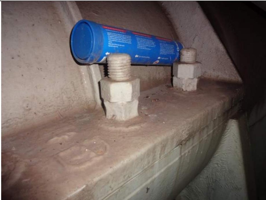
Photo 34 - [NW Outer Trunnion] – Note the section loss on trunnion bearing nuts that have been painted over.
