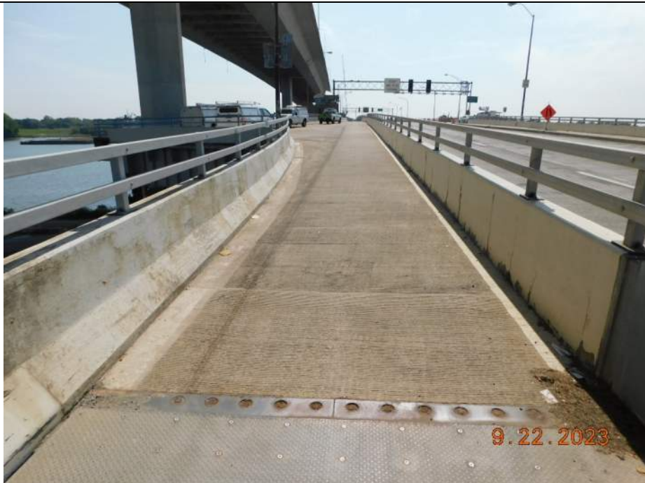
Photo S-64 - [Span 8] -Roadway deck and wearing surface, East trail, Looking South
