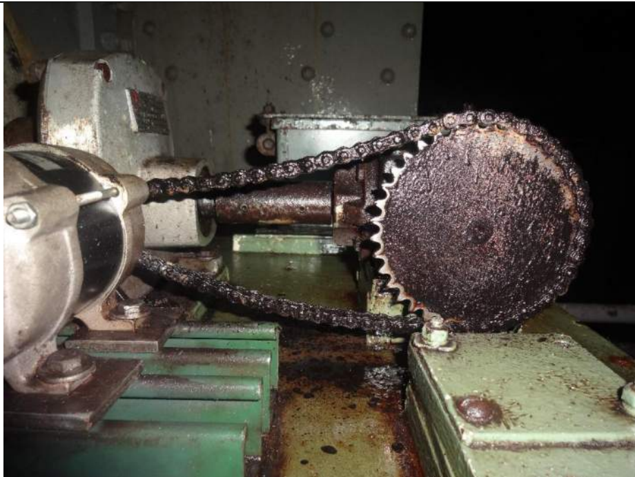
Photo 32 - [North Machinery Room] - North side span drive machinery has corrosion on shafting and loose chain.
