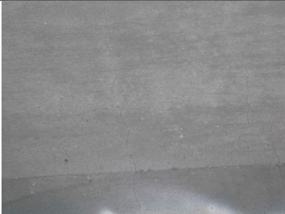
Photo S-155 - [Span 2] -Deck underside, close up view of typical 0.01-0.02" map cracking / shrinkage cracking between Floorbeams 6S & 7S, Girder 2W and Stringer 3W, Looking West
