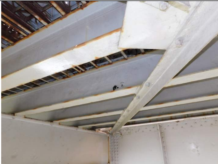
Photo S-236 - [Span 5, South Leaf] -Stringer 26W between FB4s-FB5s at mid-panel, 6" x 3" hole in web, Looking East
