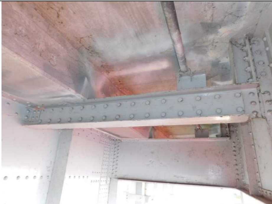
Photo S-206 - [Span 6] -Reinforcement repair to sidewalk framing member, typical, at east sidewalk between Floorbeams 1S and 2S, Looking North
