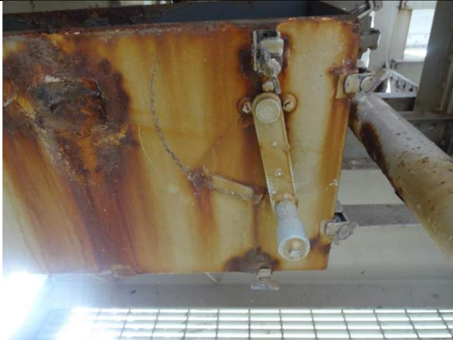
Photo 39 - [Span Lock Thruster Brake] - Span lock thruster brake lever is severely corroded and cannot be removed due to seized wingnuts.
