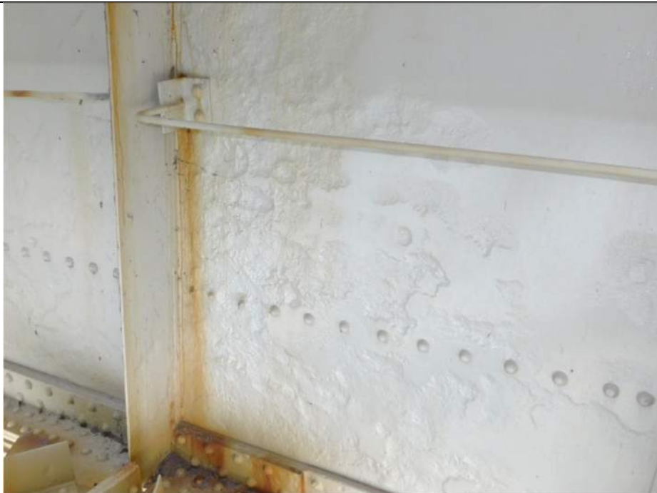
Photo S-212 - [Span 5, South Leaf] -Girder 3W, east lower web below FB5s, detail view of typical section loss up to 1/4" deep, Looking Southwest
