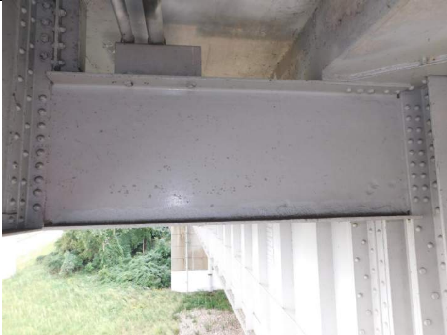
Photo S-197 - [Span 2] -Floorbeam 6S, East exterior, North face, typical painted over section loss up to 0.125" deep across lower web, Looking South
