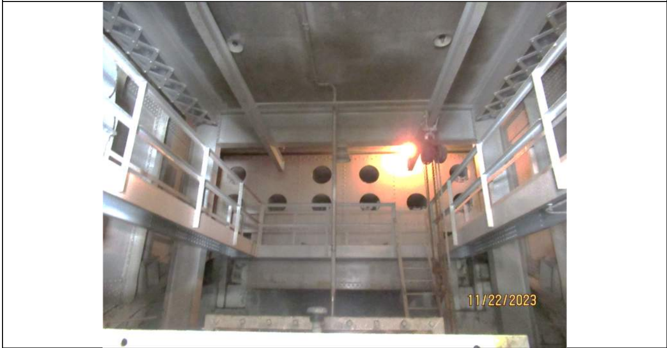
Photo S-364 - [Pier 5 Interior] -Upper catwalks between G1W and G2W in good condition, Looking North
