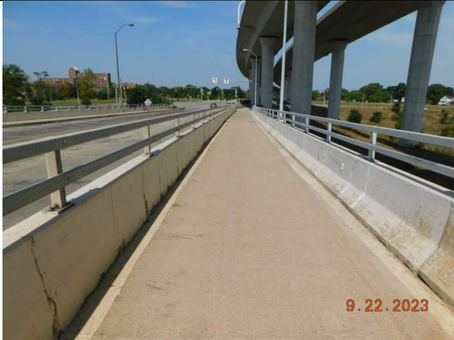
Photo S-99 - [Span 9] -East roadway & trail / sidewalk barriers and top railings, typical full height vertical cracking, Looking North
