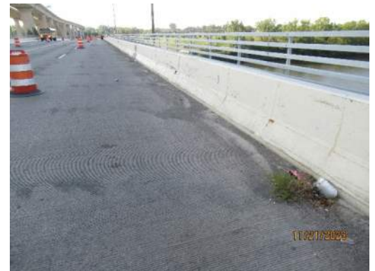
Span 3 west roadway barrier, typical cracks
