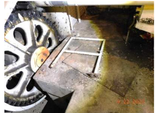
Pier 5, broken railing at machinery level
