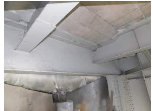
Span 4 FB36s at Pier 4, web SL and holes
