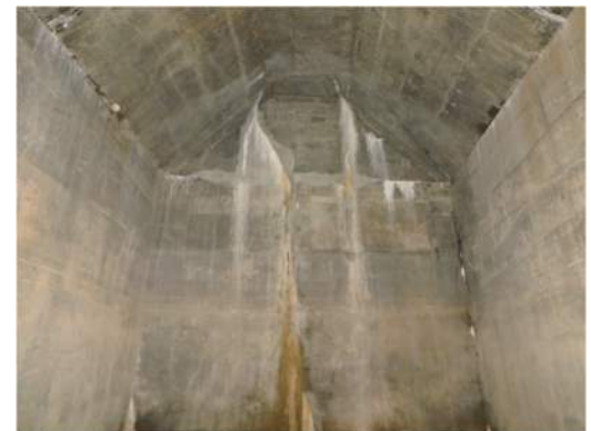
Pier 4 Basement Level F exterior wall cracks
