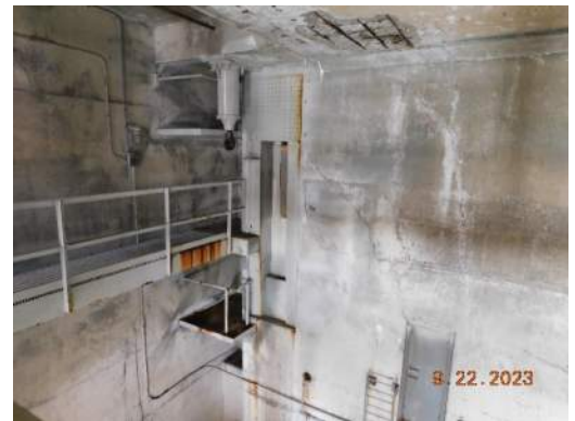
Pier 5 roadway span underside (Level C), deck spalling above G1W
