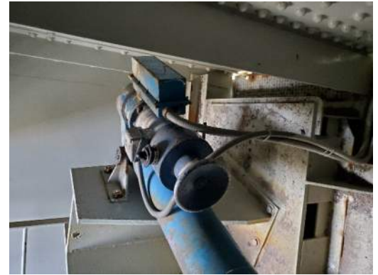
Photo E13: Southeast Traffic Gate Acuator
