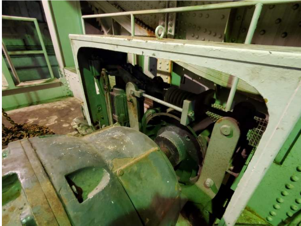
Photo E-11: Northeast Motor Brake
