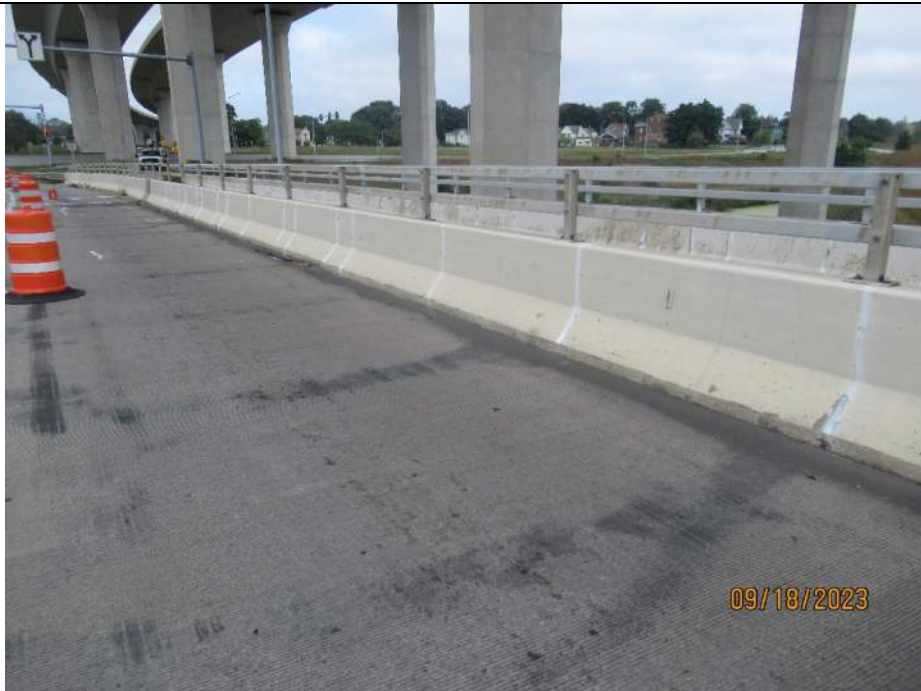
Photo S-100 - [Span 10] -East roadway barrier and top railing, trail barrier and railing in background, typical full height vertical cracking, Looking Northeast
