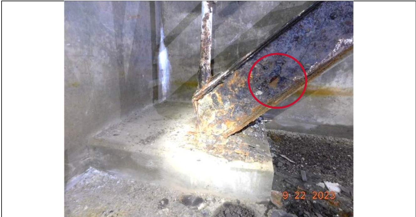
Photo S-367 - [Pier 5 Interior] -Level F, base of stairs in East exterior room, heavy corrosion, section loss, hole in channel web, Looking East
