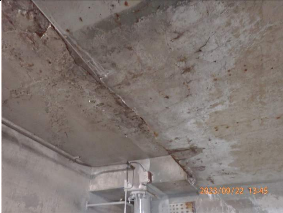
Photo S-347 - [Pier 4 Interior] -Roadway span underside (Level C) above Girder 4W, view of cracking and small spalls to deck underside above counterweight, Looking Southeast
