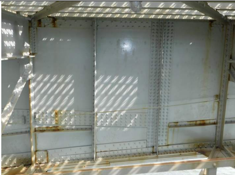
Photo S-214 - [Span 5, North Leaf] -Girder 3W, west face between FB5n-FB6n, typical scattered section loss to web and built-up components, Looking East
