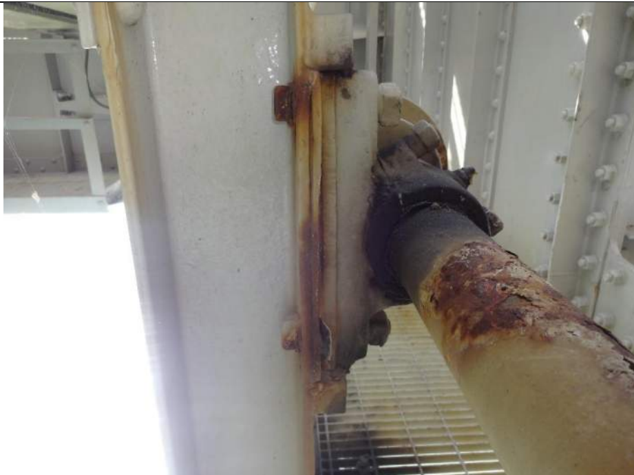
Photo 54 - [NW Span Lock Bearings] – Note pack rust forming, paint failure, isolated corrosion on fasteners on bearings.
