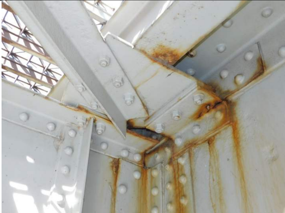
Photo S-243 - [Span 5, North Leaf] -Upper diagonal bracing at FB2n south side to G2W west side, 5" L crack in connection angle, Looking Northeast
