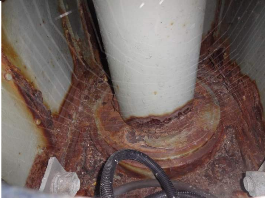
Photo 77 - [SE Swing Gate] - Heavy corrosion is on bearing and shaft inside swing gate housing.
