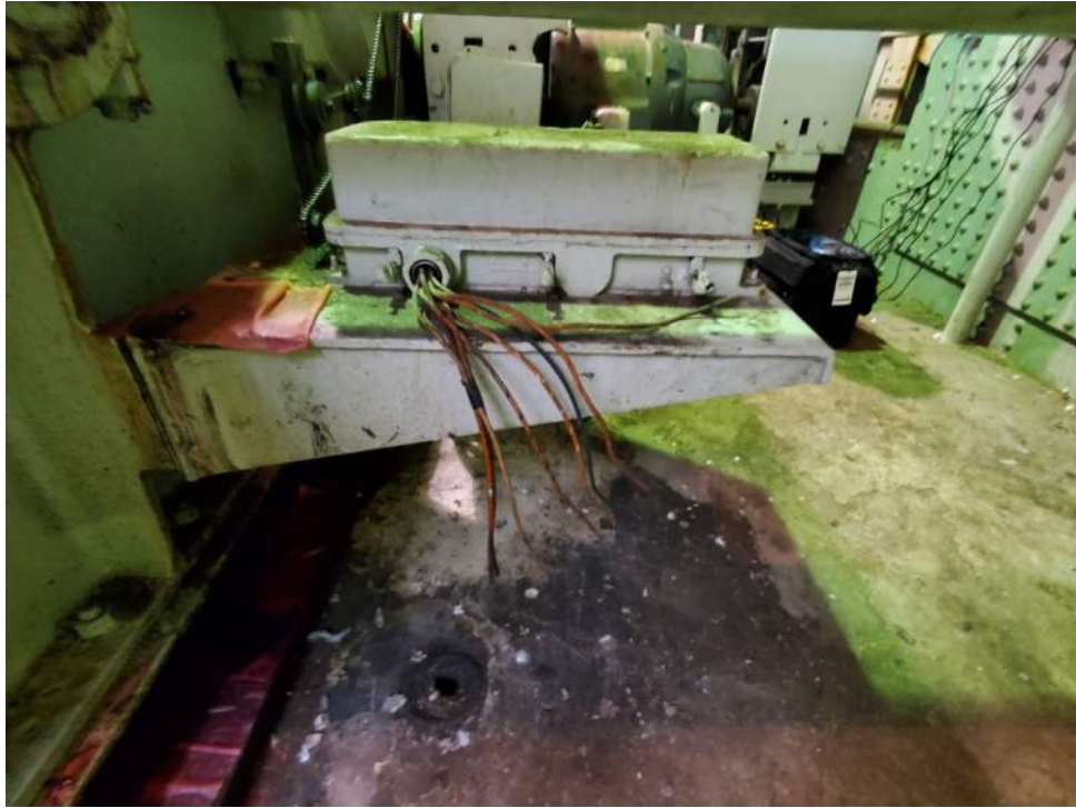
Photo E-19: Abandoned North Leaf Rotary Cam Limit Switch. Abandoned equipment should be removed
