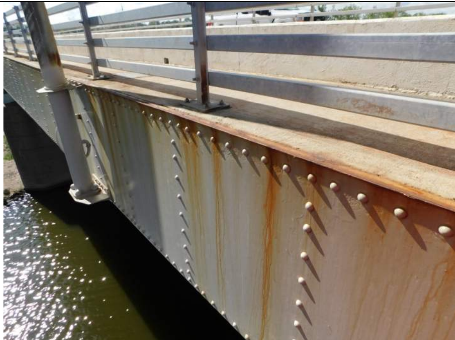
Photo S-70 - [Span 2] -East fascia, detail view of typical packing corrosion at sidewalk edge and fascia plate, Looking Southwest
