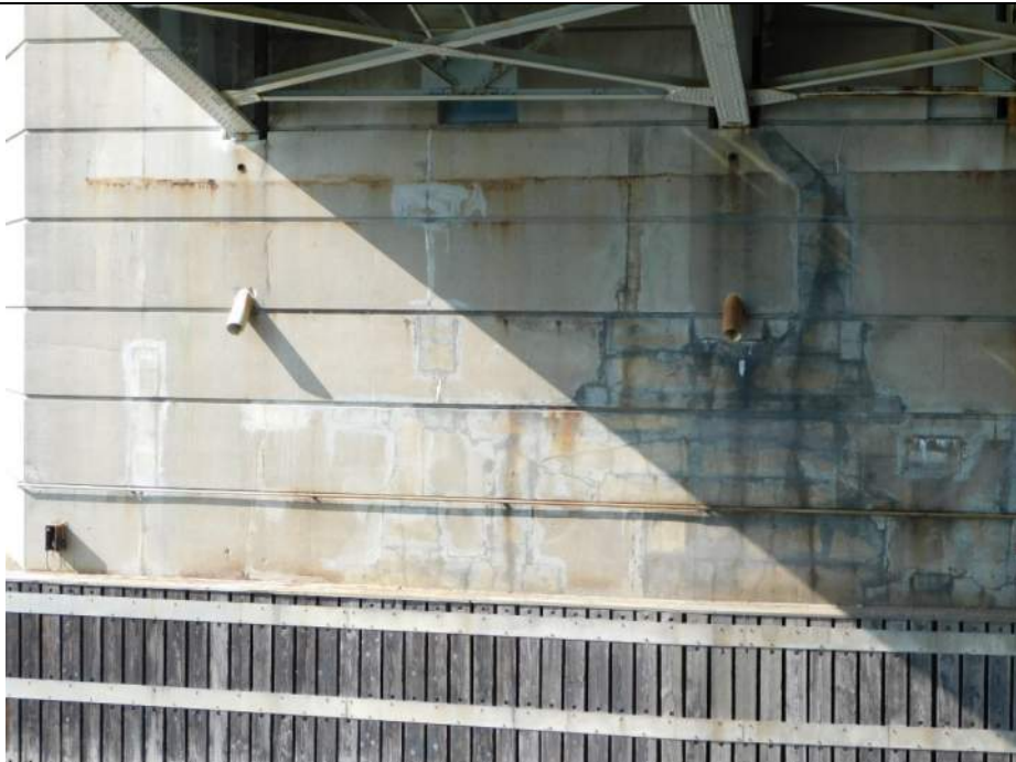
Photo S-302 - [Pier 5] -Detail view of repairs and cracking across west half of south face, Looking North
