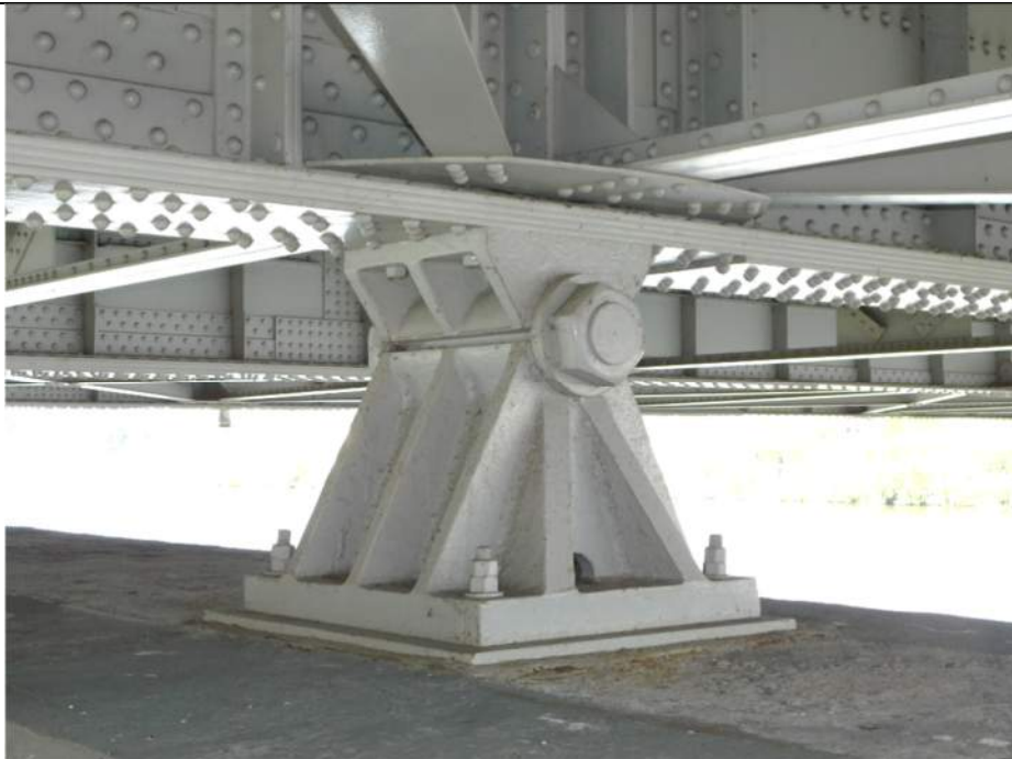
Photo S-256 - [Pier 2] -Bearing 3W general view, typical good condition of fixed bearings, Looking North
