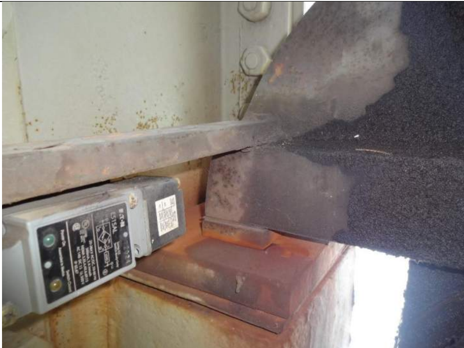
Photo 48 – [NW Inboard Locking Mechanism] – Severely corroded countersunk bolts and pack rust is forming on receiver plates.
