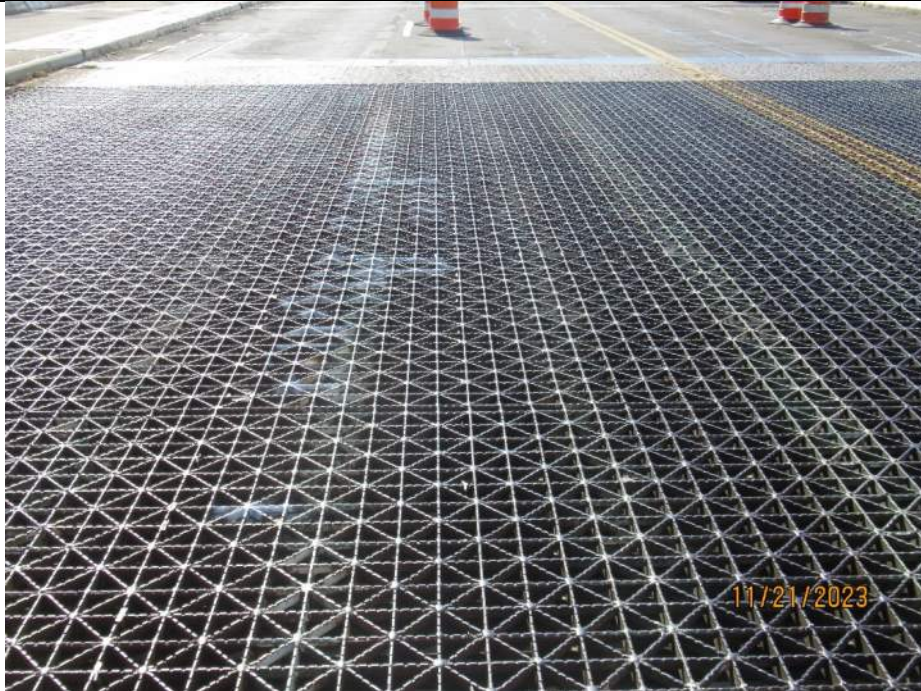
Photo S-55 - [Span 5] -South leaf, general view of grating noting locations of corrosion holes with white spray chalk, Looking South
