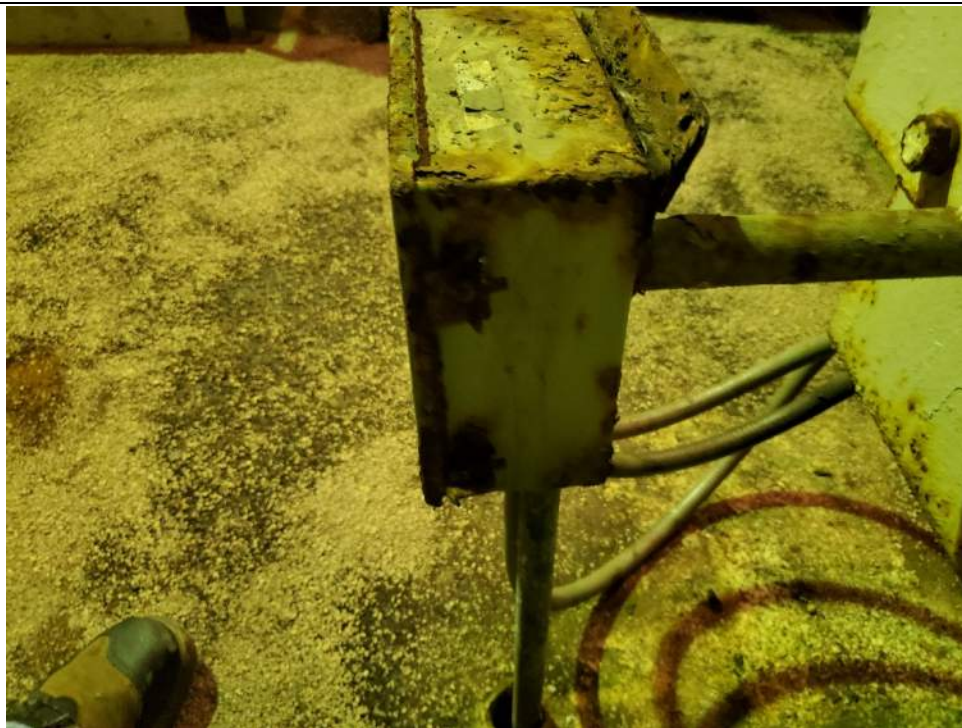
Photo E-12: Motor Brake Junction Box. Note the severe corrosion on the junction box and conduit. Also note that the junction box is not properly mounted as it is only supported by
