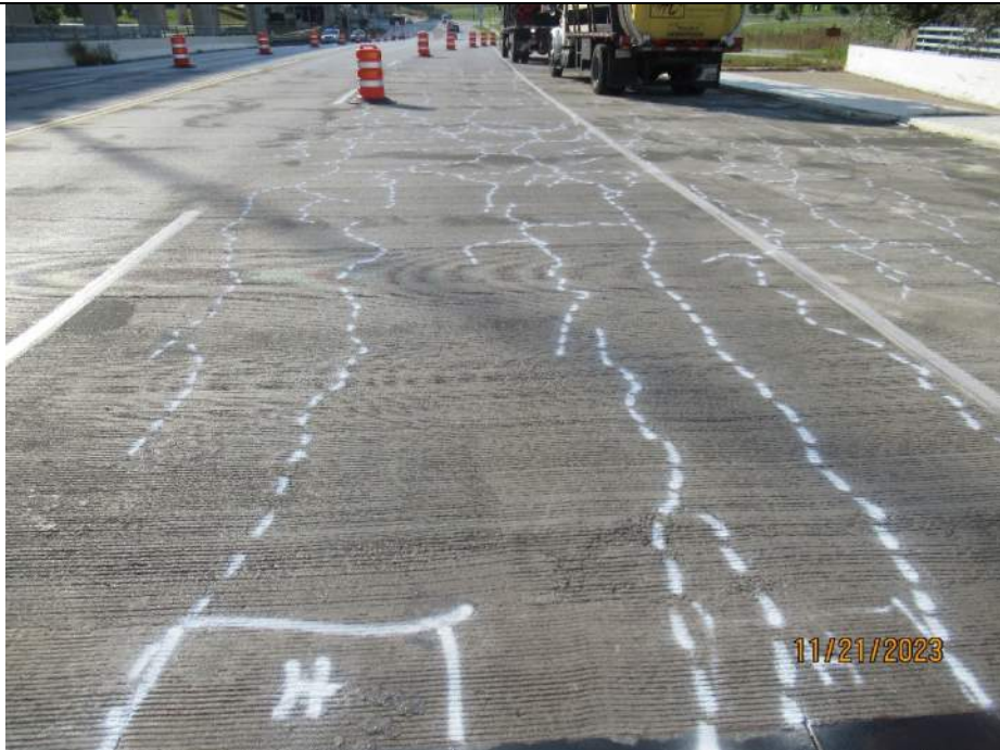
Photo S-12 - [South Approach] -Roadway approach pavement, SB lanes and shoulder general view, Looking South
