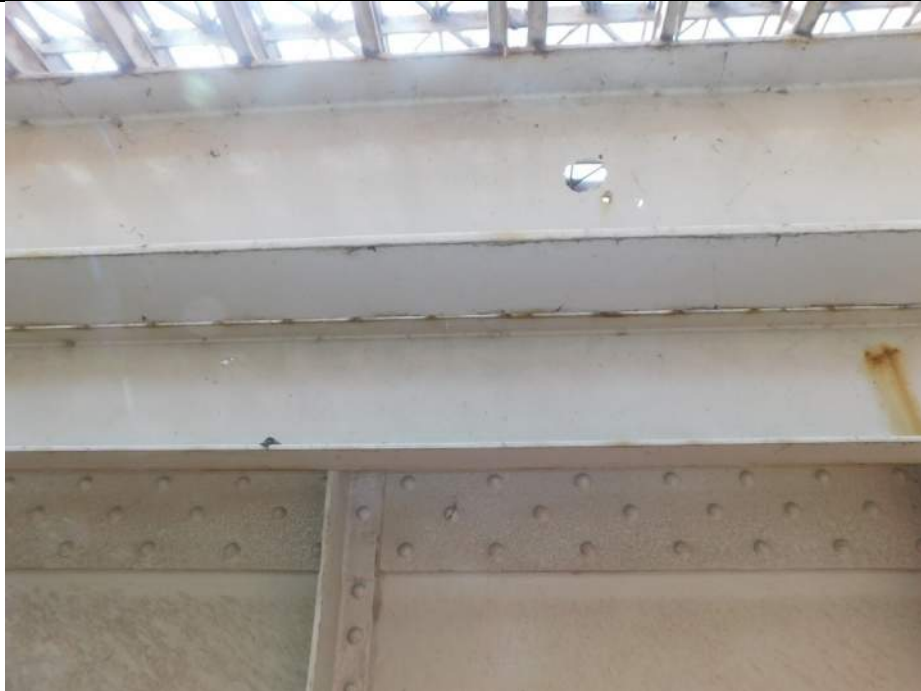
Photo S-235 - [Span 5, North Leaf] -Stringers 10W+11W at mid-panel, holes in web up to 3" diameter, Looking West
