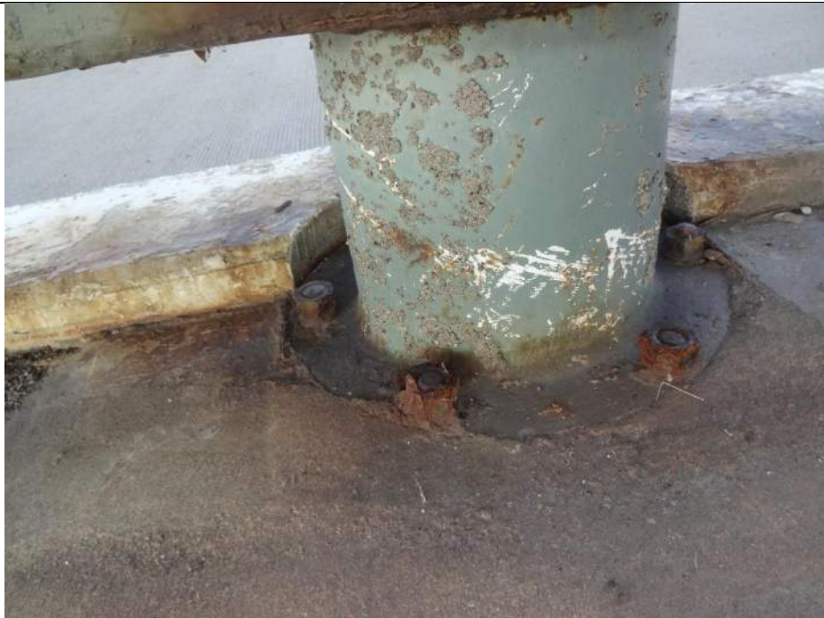
Photo 76 - [SE Swing Gate] - Severe corrosion and section loss exist on upper bearing anchors of swing gate.
