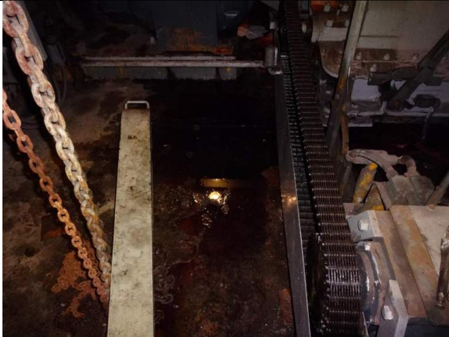
Photo 21 - [South Machinery Room] - South side gear box severely leaks oil most likely due to overfilling. Puddles of lubricant all over floor.
