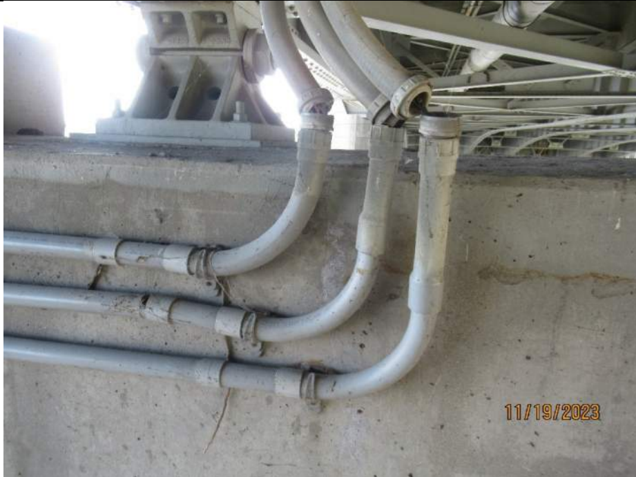
Photo S-335 - [Pier 6] -Three conduits at north face of pier are disconnected with exposed wiring, Looking South
