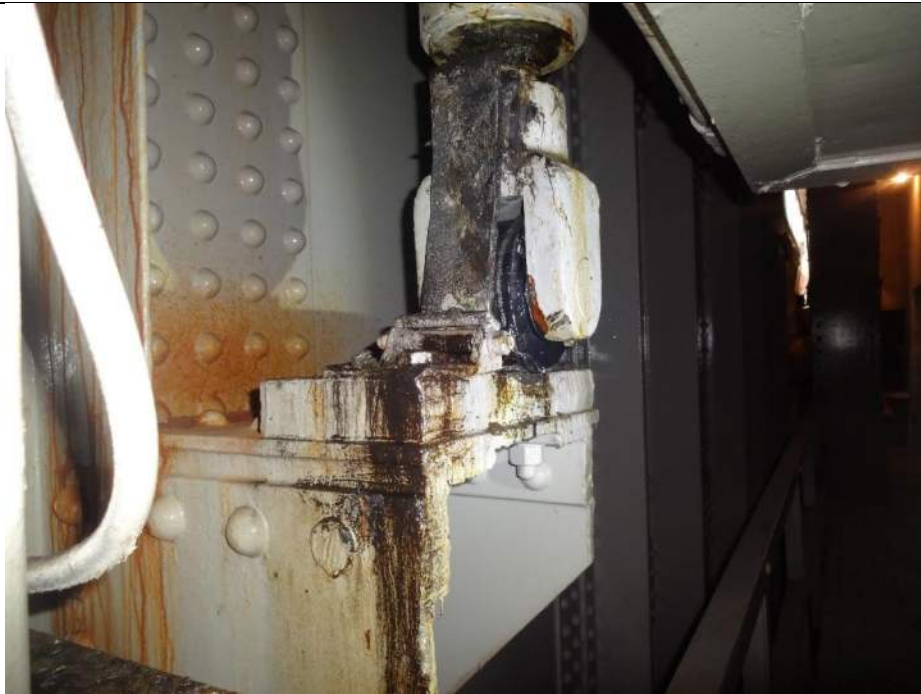
Photo 58 - [SE Seated Buffer] - Seated buffer has moderate grease purge.
