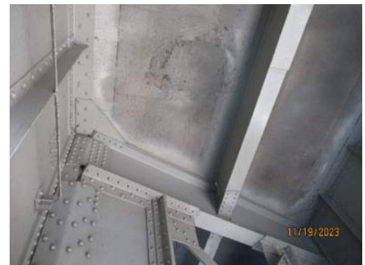
Span 7 deck underside typical patch repair
