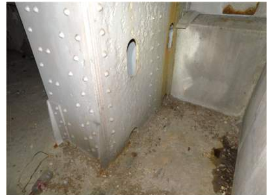
Pier 4 Trunnion Tower 4W, West leg base, exterior plate section loss
