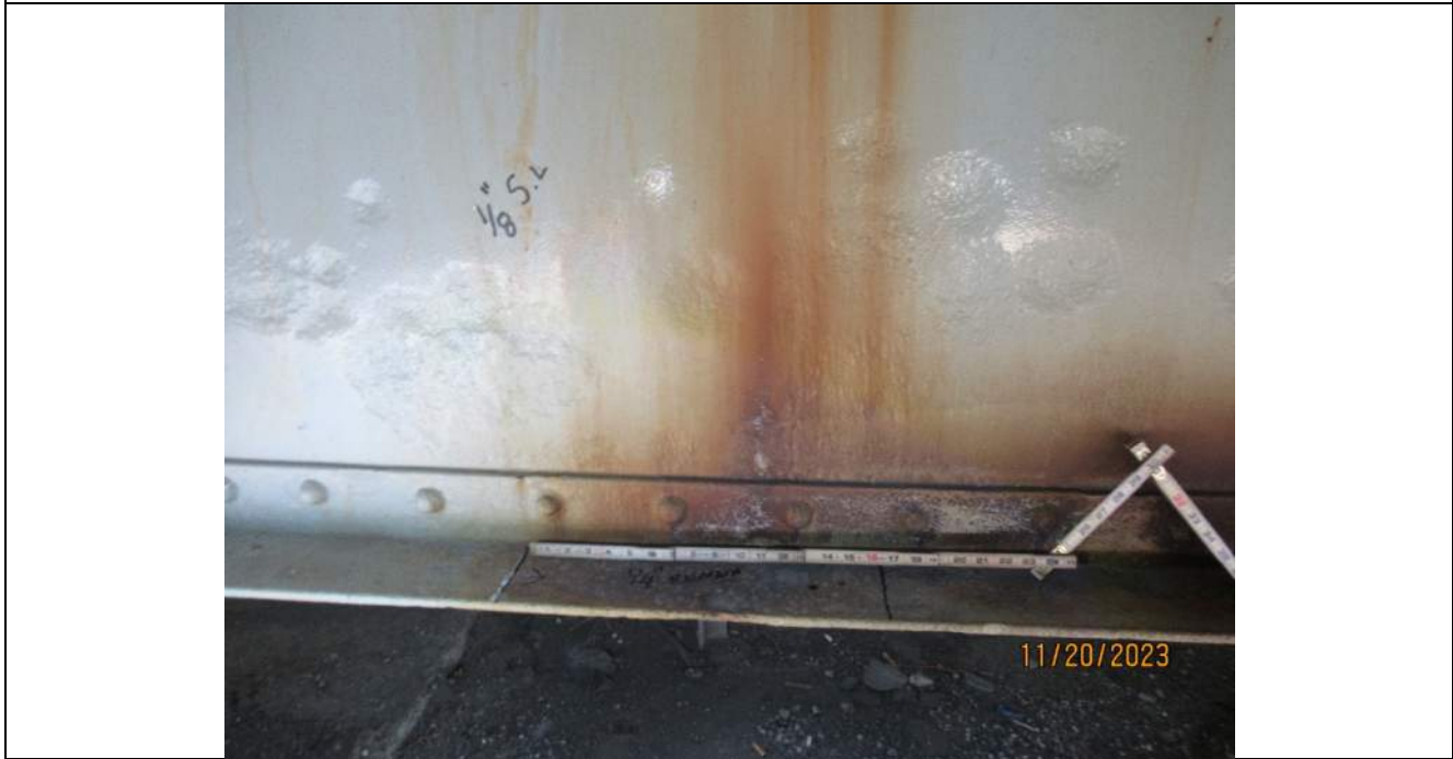
Photo S-192 - [Span 8] -Floorbeam 20S, south lower web and bottom flange between G2W-G3W, typical scattered web section loss and localized section loss at bottom flange, Looking North
