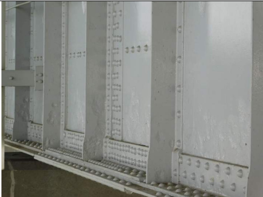
Photo S-180 - [Span 4] -Girder 4W East lower web between FB28S-29S exhibits typical scattered painted over section loss to lower web up to 0.125" deep, Looking Southwest
