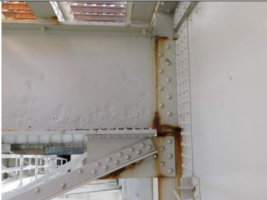
Photo S-242 - [Span 5, South Leaf] -K-bracing below FB4s between G2W-G3W, 1" dia hole in connection plate, Looking South (note typical PR and SL to FB web & connection)
