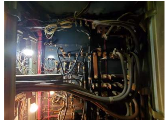
Photo E7: Back Side of the South Leaf Motor Starter Cabinet
