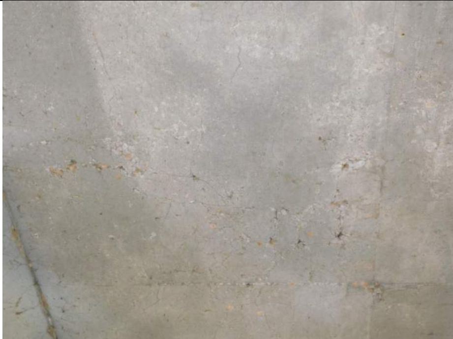
Photo S-157 - [Span 2 ] -Deck underside, between Floorbeam 14S-15S and Stringers 5W-6W, typical minor map cracking and honeycombing, Looking South
