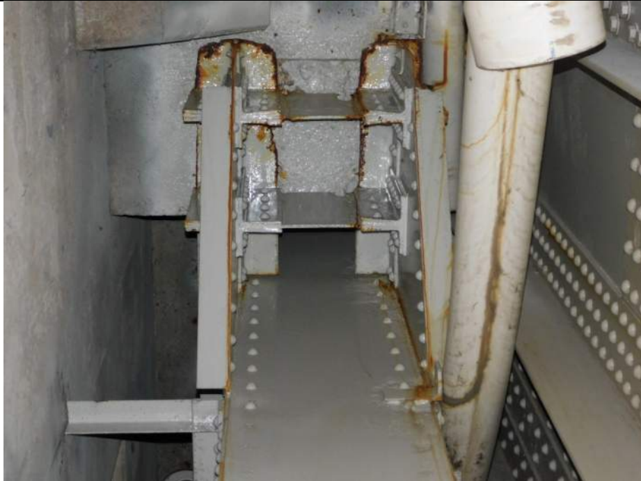
Photo S-355 - [Pier 4 Interior] -Tower 4W East leg North column at trunnion pin access catwalk location, North side framing exhibits 100% edge section loss, Looking South
