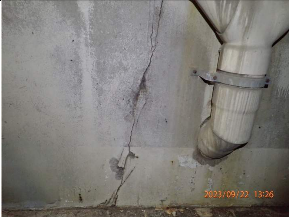
Photo S-345 - [Pier 4 Interior] -Machinery level (Level D) channel side wall between Girders 3W and 4W, wide vertical crack behind drainage pipe, Looking North
