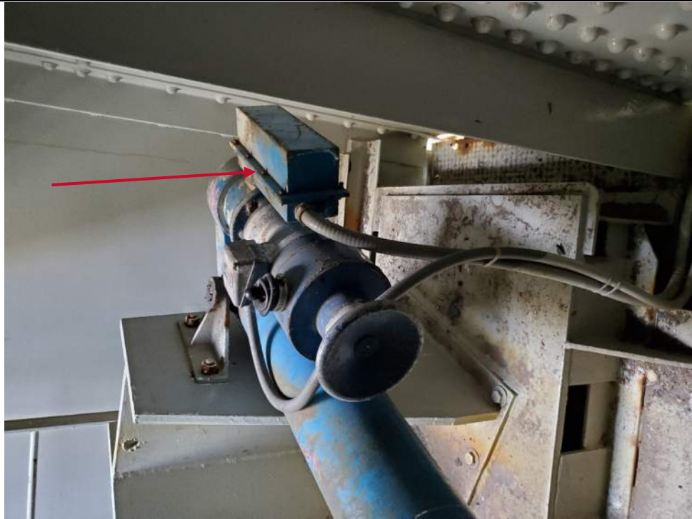
Photo E-13: Southeast Traffic Gate Actuator. Note the corrosion and the abandoned in place rotary cam limit switch.
