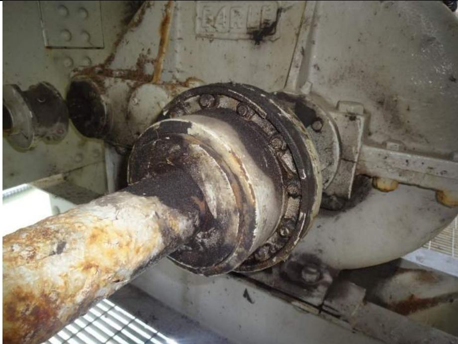
Photo 45 - [NW Span Lock Couplings] - Couplings exhibit minor paint failure, moderate grease purging, and rusted hubs.
