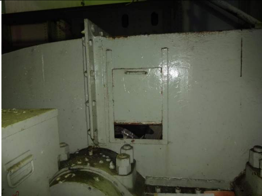
Photo 19 - [North Machinery Room] - Inspection hatches on central gear enclosure do not fully open due to being painted over.
