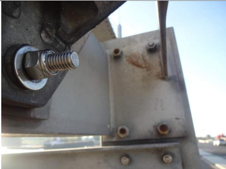
Photo 64 - [NE Traffic Gate] - Cracked welds are at base of gate arm and isolated corrosion is present on fasteners of arm connector.
