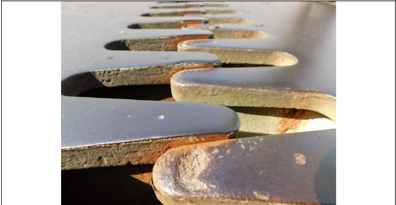
Photo S-140 - [Span 5] -Bascule span center finger joint, detail view of horizontal mis-alignment with fingers in contact, Looking East
