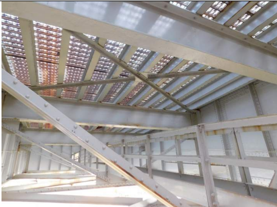
Photo S-270 - [Span 5, South Leaf] -Stringers, floorbeams, bracing and catwalk between G2W-G3W and FB5s-6s-7s, general view of paint in good condition, Looking North
