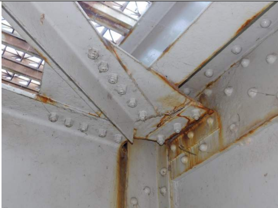
Photo S-238 - [Span 5, South Leaf] -Upper diagonal bracing at FB6s south side to G2W west side, connection angle fully cracked/broken, Looking Northeast
