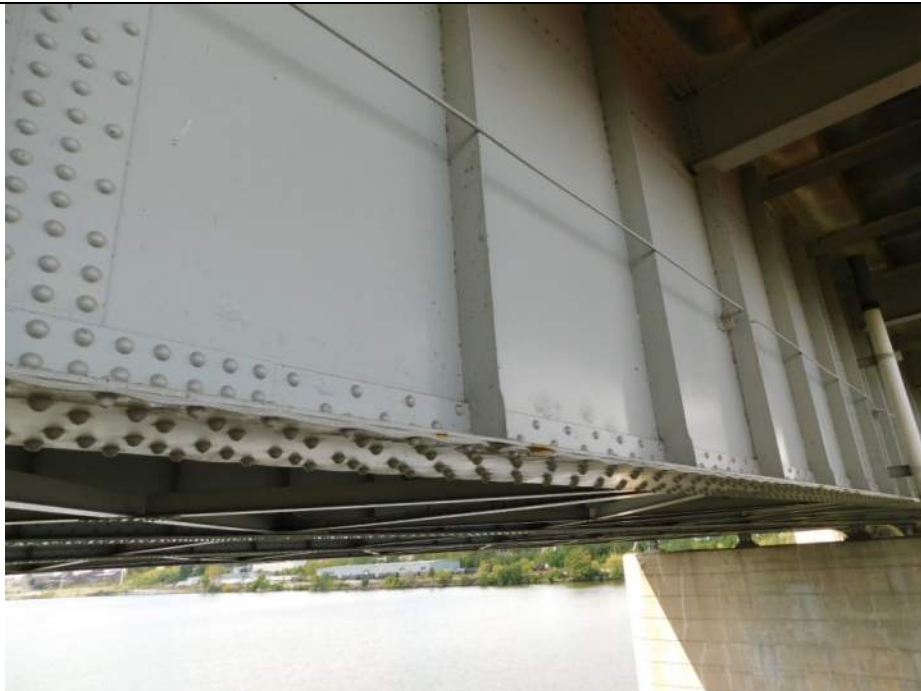
Photo S-178 - [Span 3] -Girder 4W East bottom flange, warping of cover plates due to packing corrosion, general view, Looking Northwest
