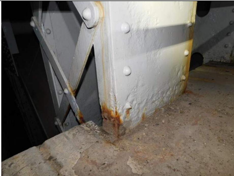
Photo S-354 - [Pier 4 Interior] -Tower 4W East leg at machinery level, section loss and hole in North column North channel, Looking Southwest
