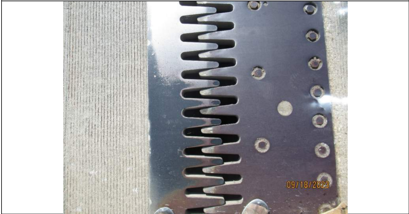
Photo S-122 - [South Abutment] -Abutment reference line finger joint, horizontal mis-alignment with fingers touching in NB lanes, Looking West
