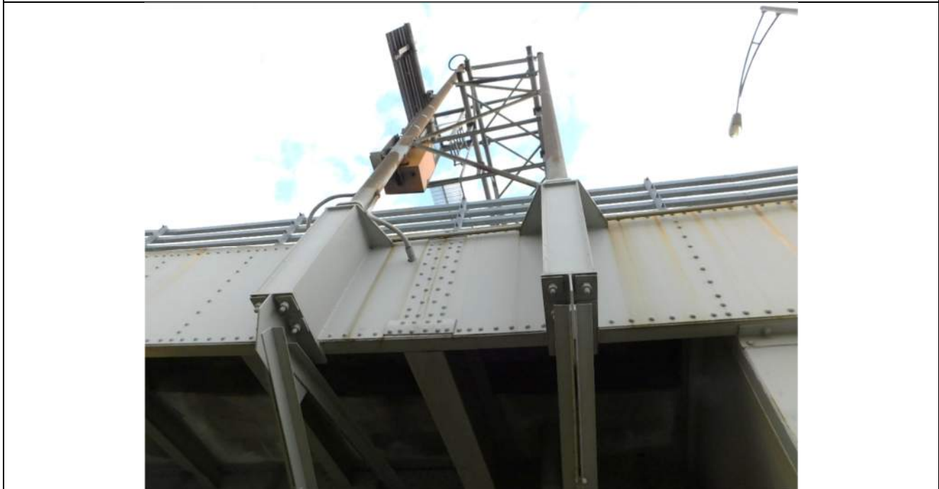
Photo S-330 - [Span 6] -Sign gantry support connections at West fascia, posts and bases in good condition, Looking East
