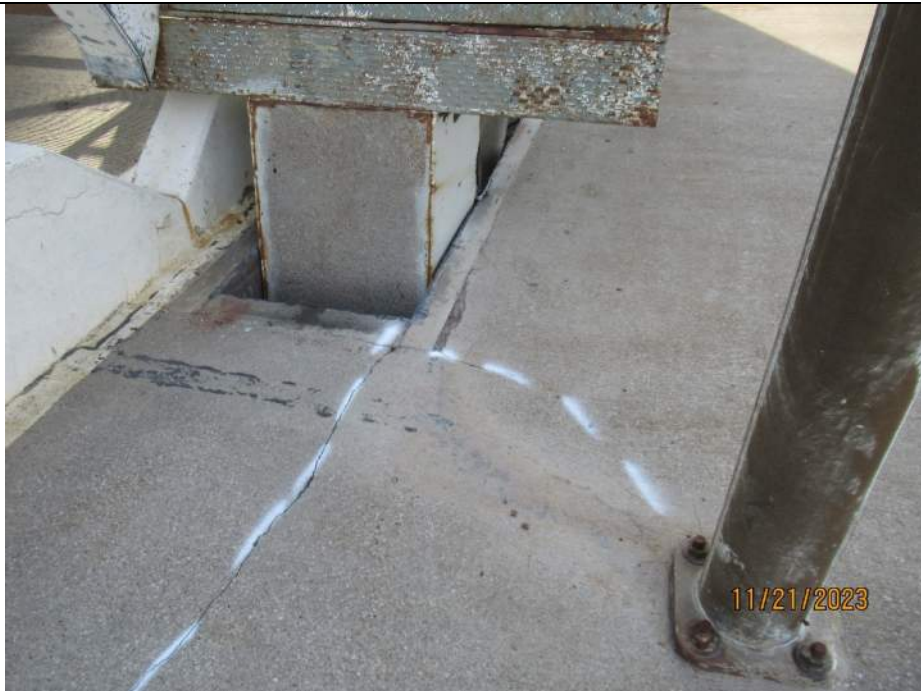
Photo S-144 - [Pier 5] -North rear break joint at Girder 1W longitudinal break, slight rubbing/wear between break edge angles and girder cap vertical plates, Looking South
