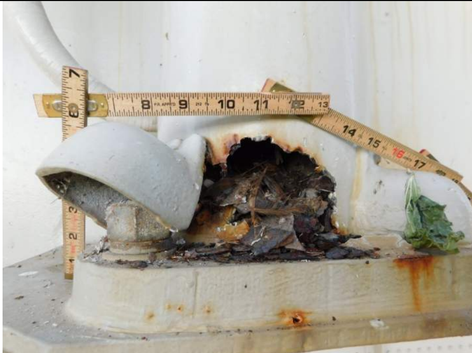
Photo S-316 - [Span 1] -East side light pole at Floorbeam 4S, holes in base of pole at west and north sides up to 6" W x 4" H, Looking West
