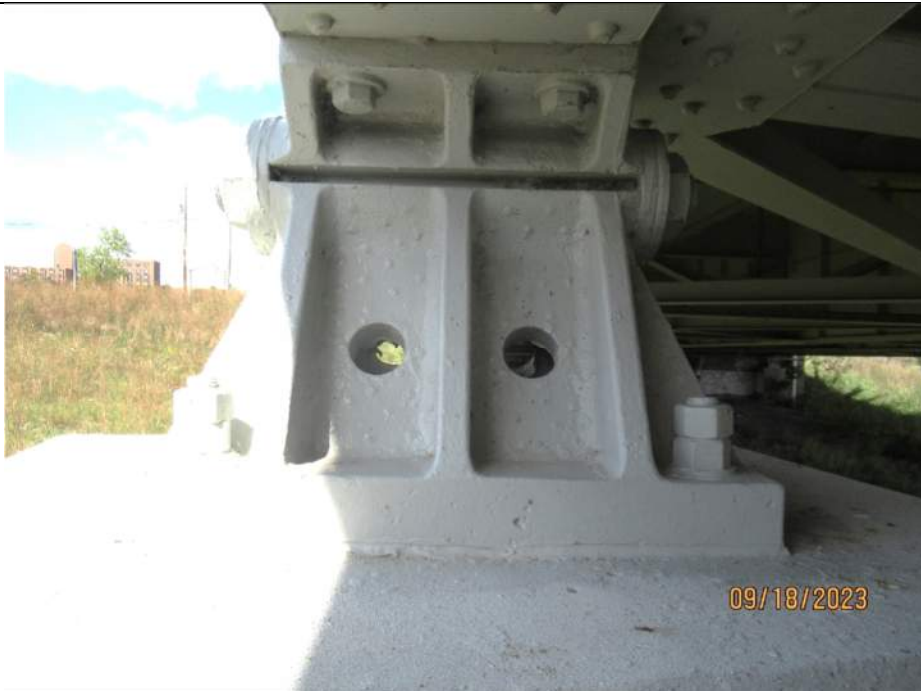
Photo S-268 - [Pier 9] -Bearing 1W, fixed bearing in good condition, typical for Pier 9 fixed bearings, Looking North
