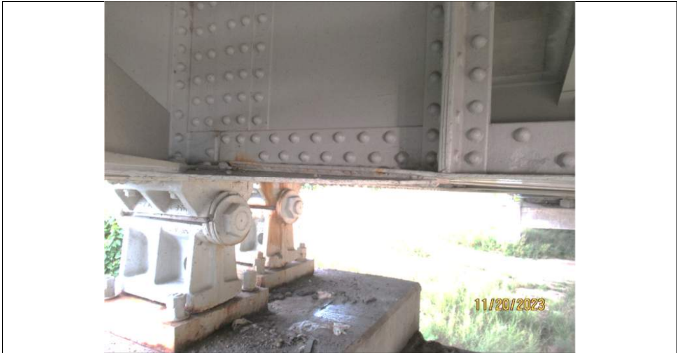
Photo S-191 - [Span 8] -Floorbeam 20S south bottom flange, pack rust and warping of flange angle at the lower diagonal connection plate, Looking North
