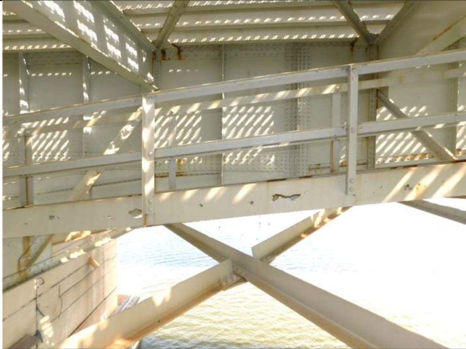
Photo S-253 - [Span 5, North Leaf] -Middle catwalk, west support channel exhibits several large holes in the web between FB5n-FB6n, Looking East
