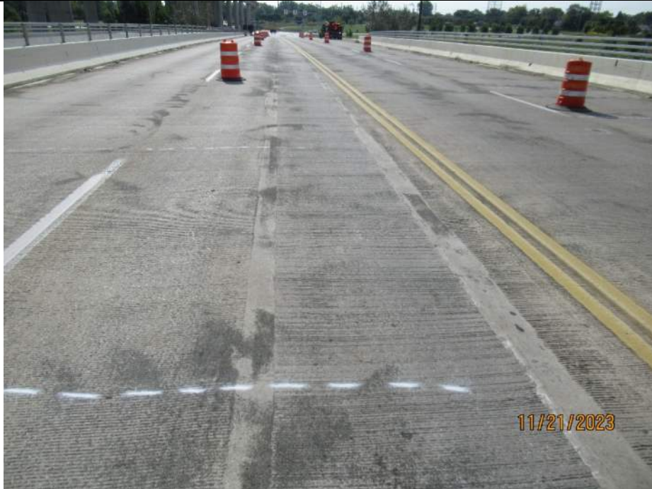
Photo S-41 - [Span 2] -Roadway deck and wearing surface, middle lanes from north end of span, Looking South
