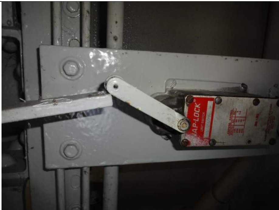
Photo 74 - [SE Swing Gate] - Limit switches have seized rollers due to paint and make poor contact with their targets.
