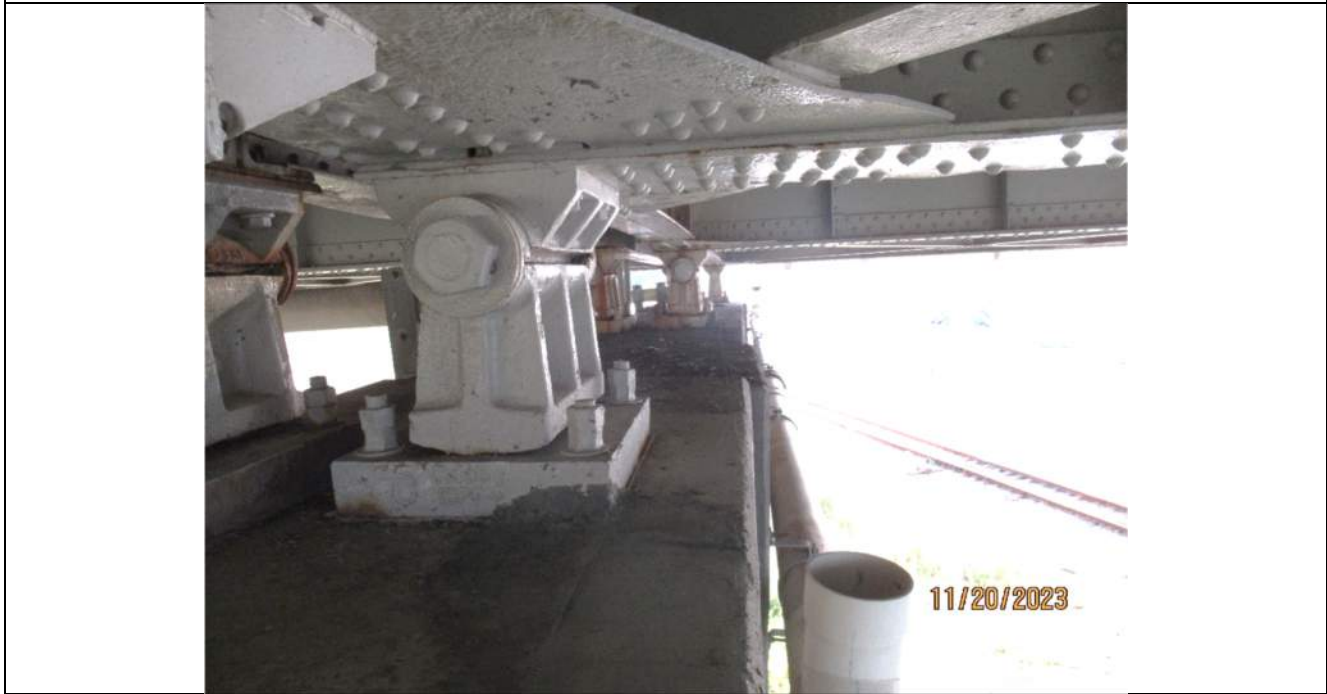
Photo S-266 - [Pier 8] -Bearings 2W, 3W, 4W (Span 8 side), minor to moderate blistering and bleeding corrosion, debris across pier top, Looking East
