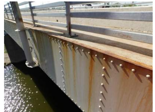
Span 2 East fascia packing corrosion
