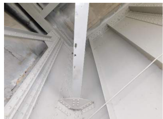
Span 4 lower diagonal to G2W flange holes
