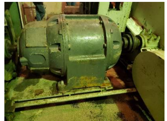
Photo E9: Southeast Main Drive Motor
