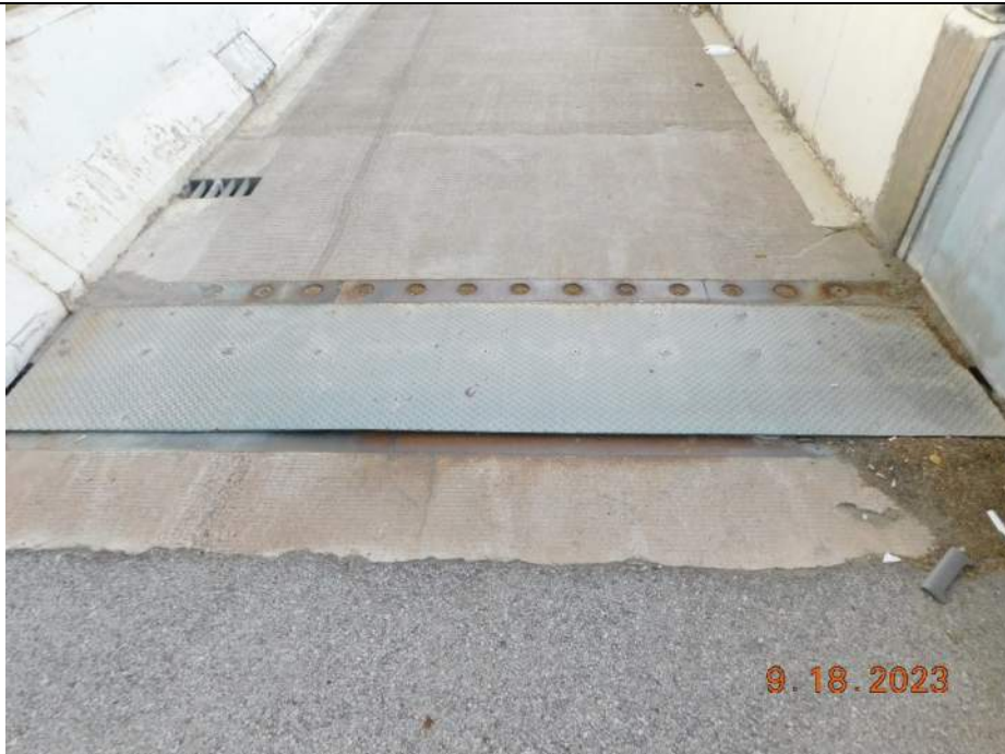
Photo S-132 - [North Abutment] -Abutment reference line finger joint with cover at east sidewalk / trail, Looking South
