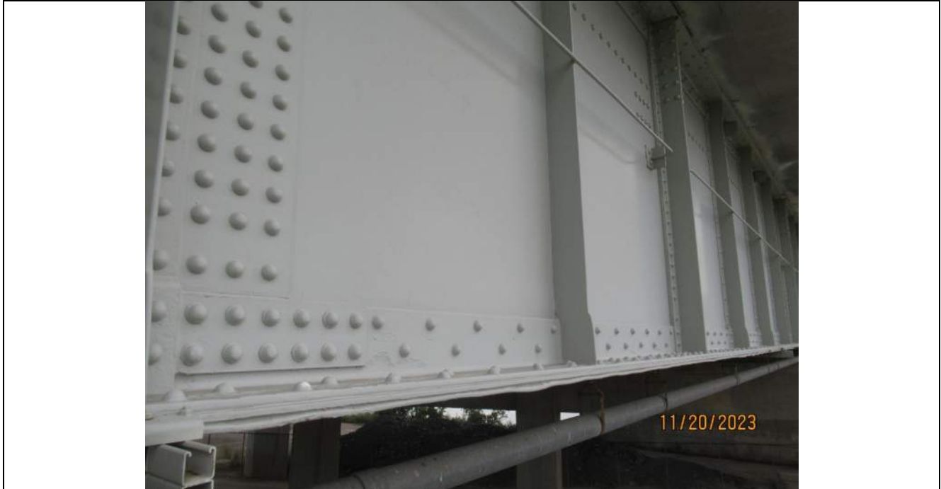
Photo S-183 - [Span 8] -Girder 1W West bottom flange, warping of cover plates due to packing corrosion, general view, Looking Southeast
