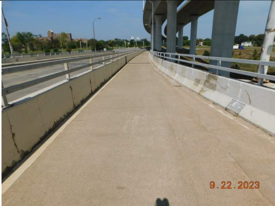
Photo S-97 - [Span 8] -East roadway & trail / sidewalk barriers and top railings, typical full height vertical cracking, Looking North
