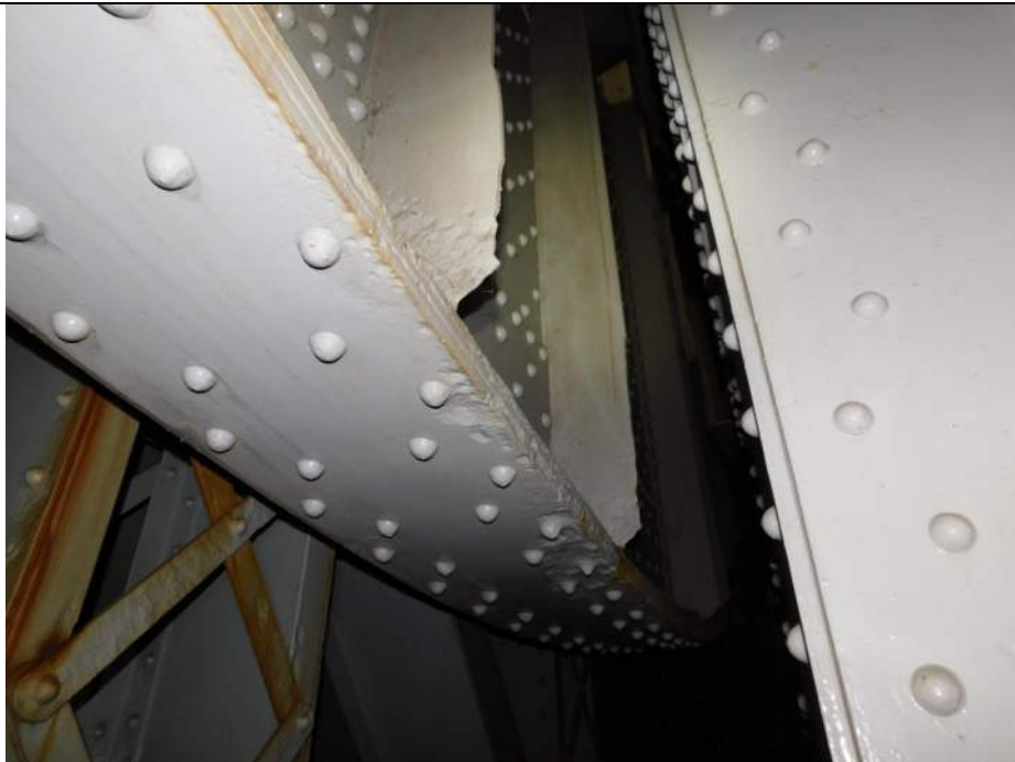
Photo S-356 - [Pier 4 Interior] -Girder 4W, West bottom flange and stiffener bases exhibit localized section loss, Looking Southeast
