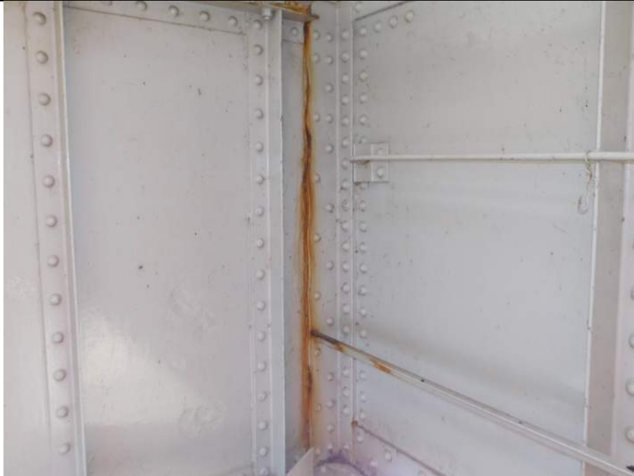
Photo S-227 - [Span 5, North Leaf] -Floorbeam 1n at east side G2W, typical packing corrosion with warping at connection angle, Looking South
