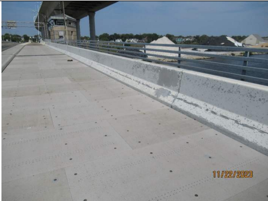
Photo S-92 - [Span 5] -South leaf, East roadway / trail steel barrier, generally good condition with flaking and peeling paint, Looking Northeast
