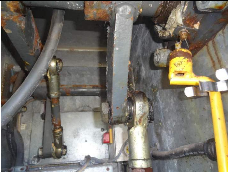
Photo 66 - [NE Traffic Gate] - Widespread corrosion and paint failure is present across all movable components.
