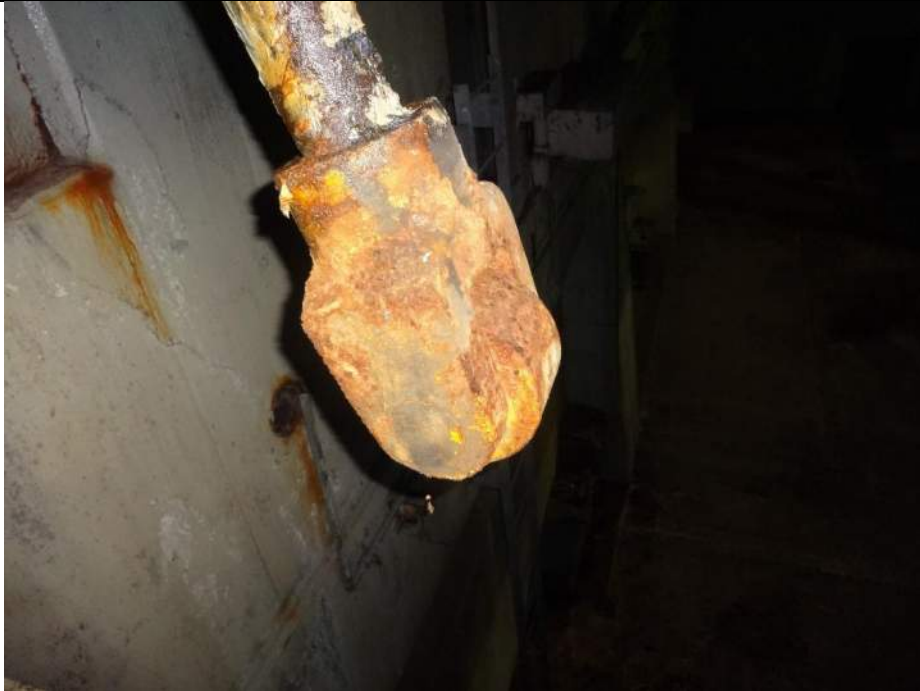
Photo 59 - [NW Raised Buffer] - Rollers of raised buffers are severely corroded and seized.
