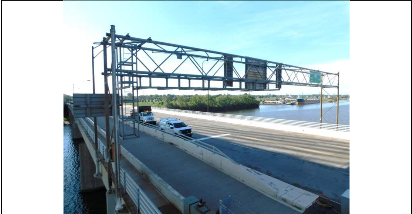
Photo S-328 - [Span 4] -Overhead Sign Gantry, general north elevation view from east side, Looking Southwest
