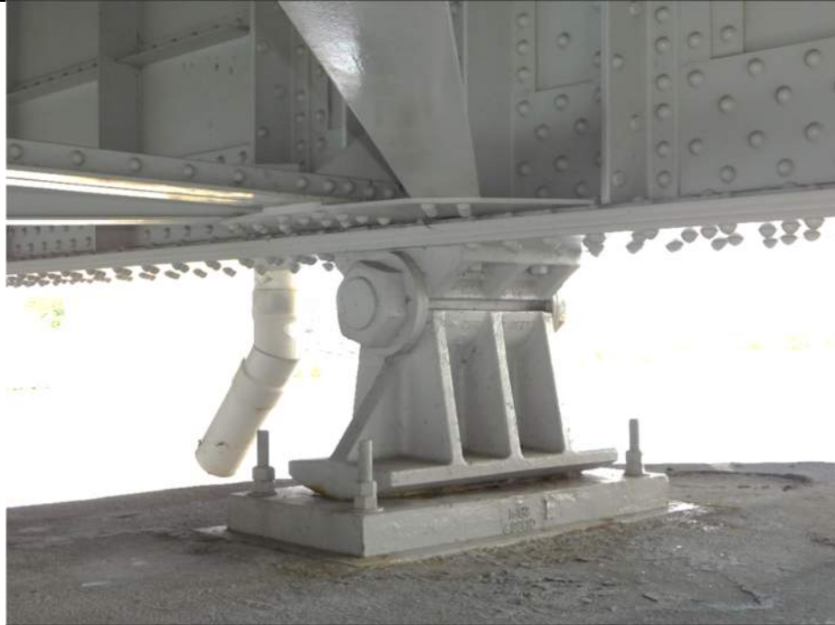
Photo S-257 - [Pier 3] -Bearing 4W general view, typical minor tilt to south in contraction, good condition, Looking Northeast
