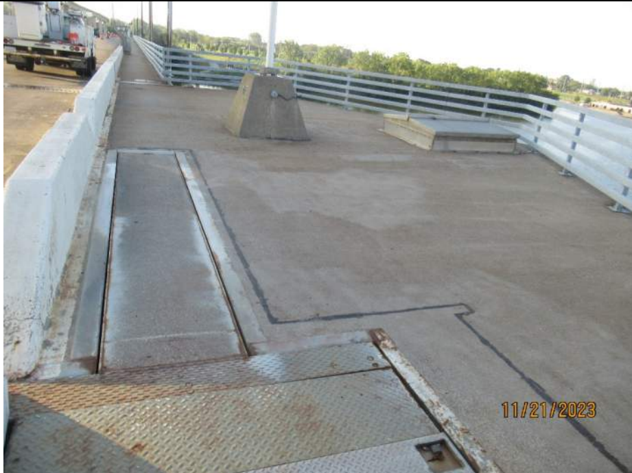
Photo S-106 - [Pier 4 Span] -West sidewalk and railings, good condition general view, Looking Southwest
