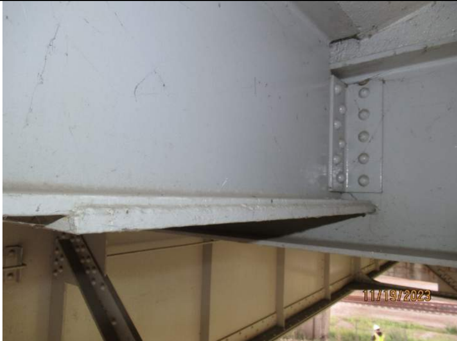
Photo S-202 - [Span 9] -Stringer 3W at connection to Floorbeam 3S, typical welded bottom flange connection plate, connection, and components in good condition, Looking South
