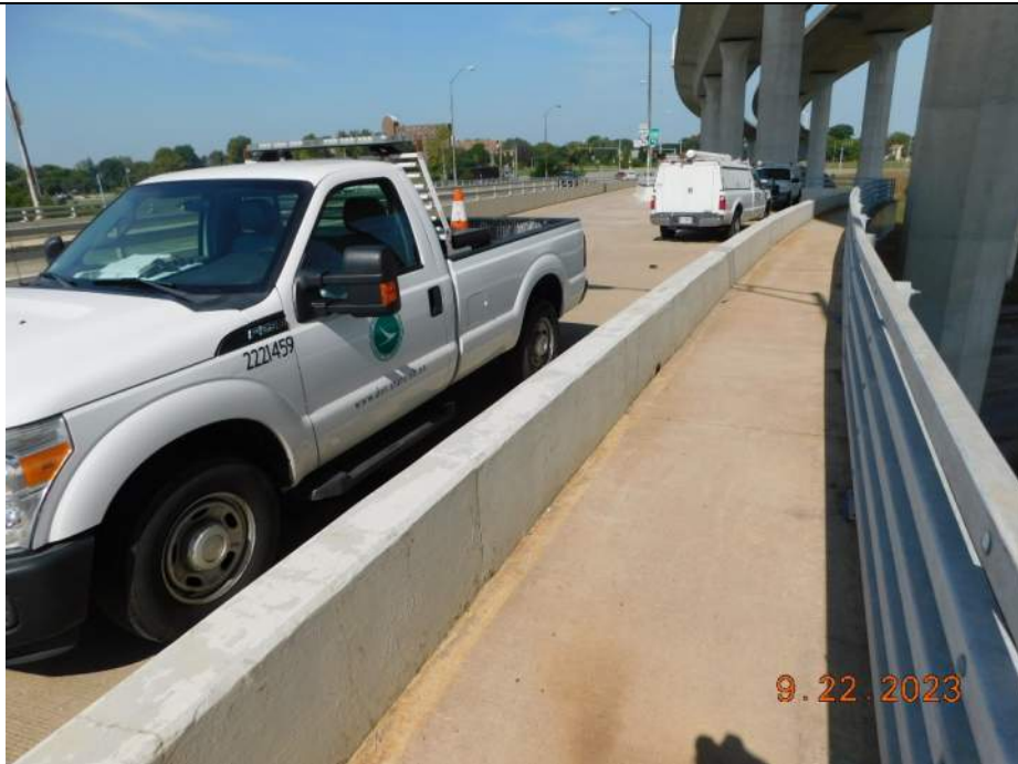
Photo S-116 - [Span 7] -East sidewalk, railing and barrier, good condition general view, Looking North
