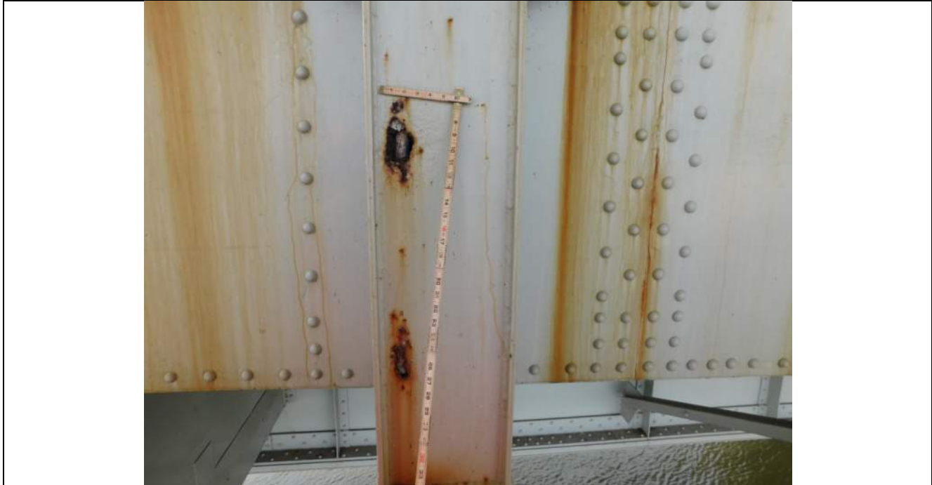
Photo S-329 - [Span 6] -Sign gantry support connection at East fascia, south post base exhibits two corrosion holes in the east plate up to 4" x 2", Looking West
