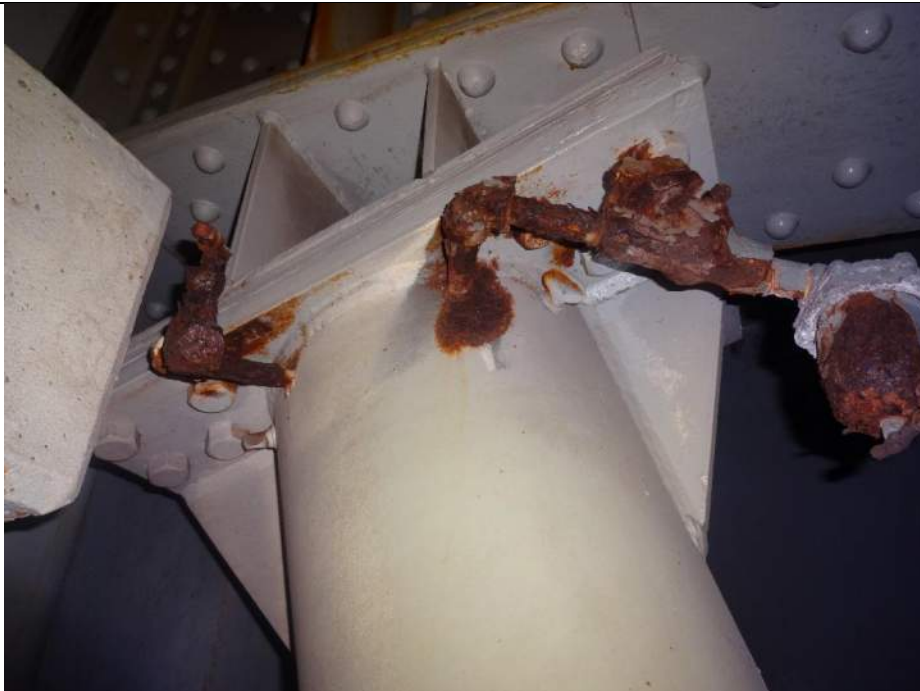
Photo 60 - [NW Raised Buffer] - Relief valves on North side of bridge are severely corroded on raised buffers.
