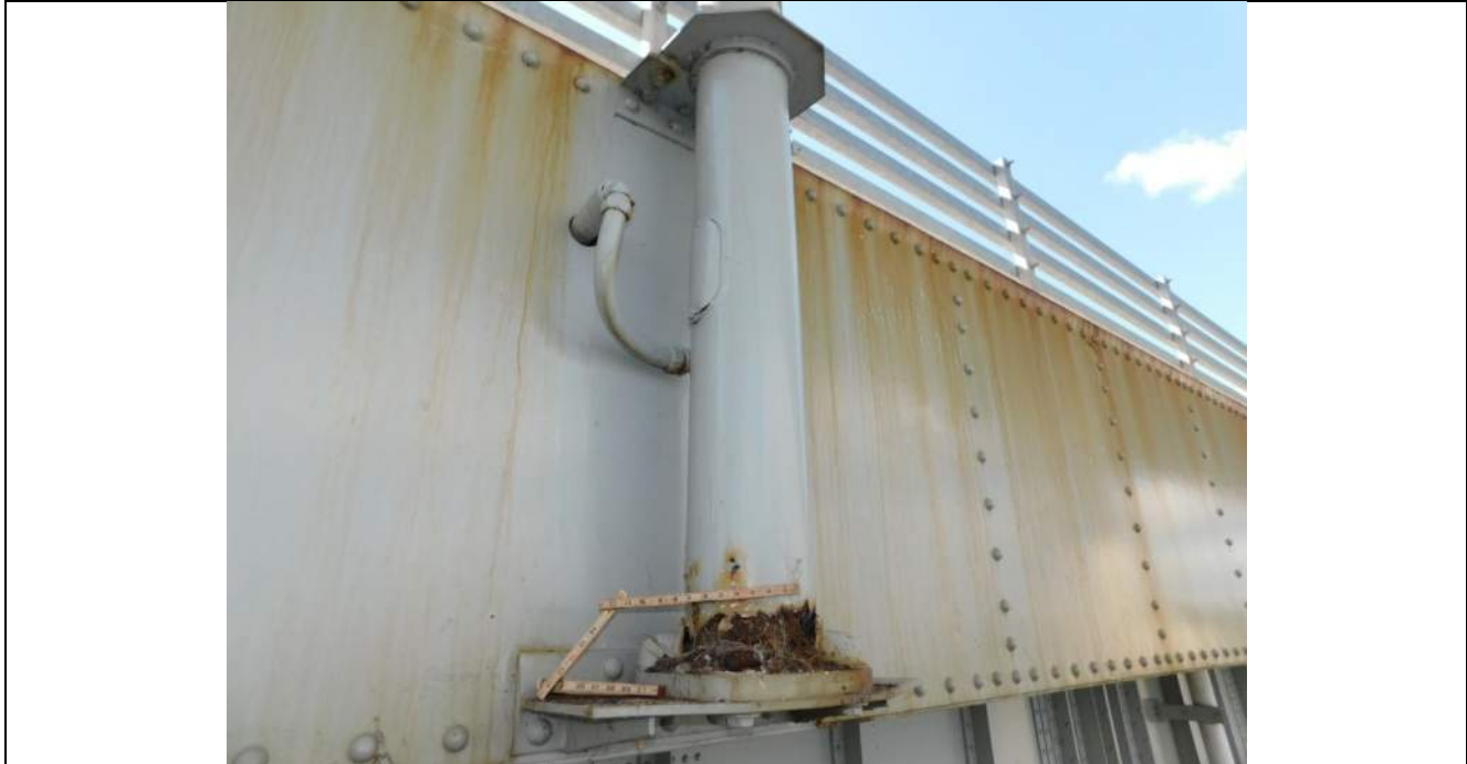
Photo S-319 - [Span 3] -East side light pole at Floorbeam 25S, holes in base of pole around 75% of perimeter, general view, Looking North
