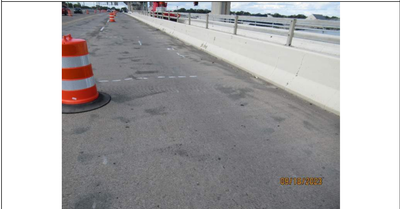
Photo S-86 - [Span 3] -East roadway barrier, typical full height vertical cracking, Looking East
