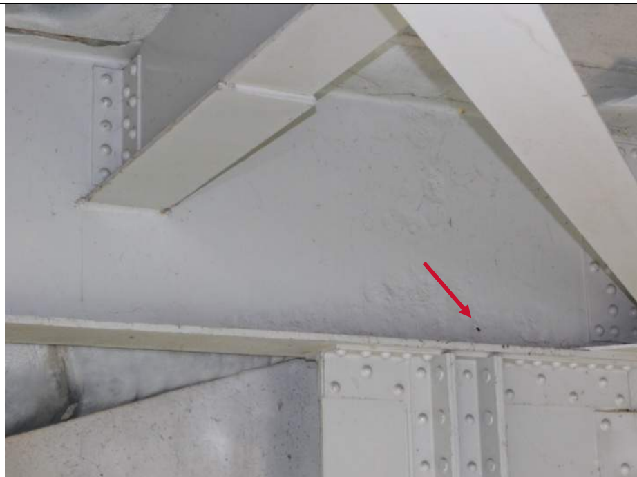
Photo S-188 - [Span 4] -Floorbeam 36S at Pier 4 between Girders 1W and 2W, painted over section loss at lower web with a small hole, Looking Northeast
