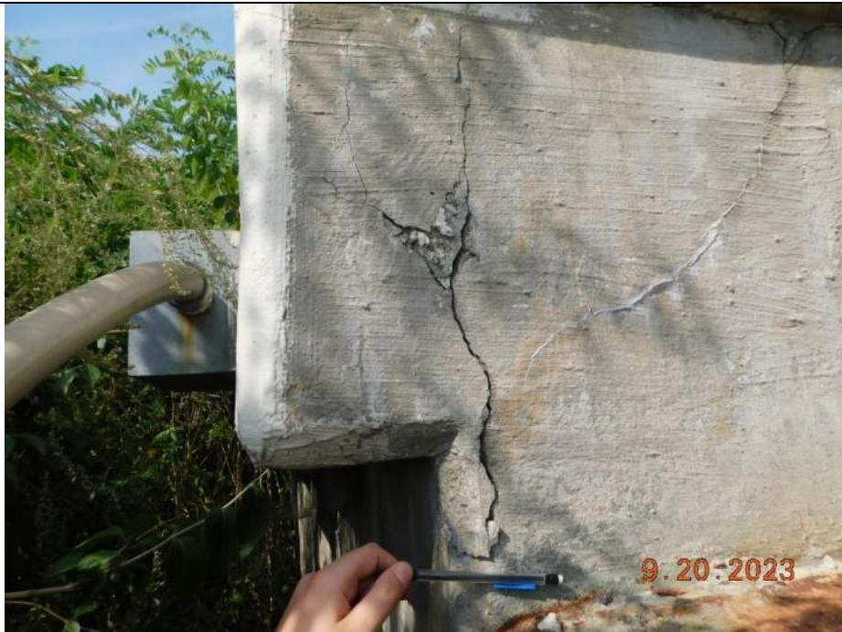
Photo S-282 - [North Abutment] -West side of backwall at West wingwall, vertical cracking at wall corner, Looking North
