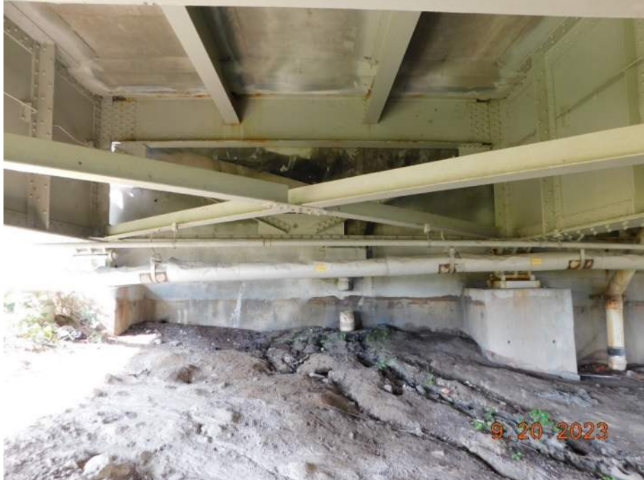
Photo S-279 - [North Abutment] -Abutment columns and back wall view between Girders 1W and 2W, Looking North
