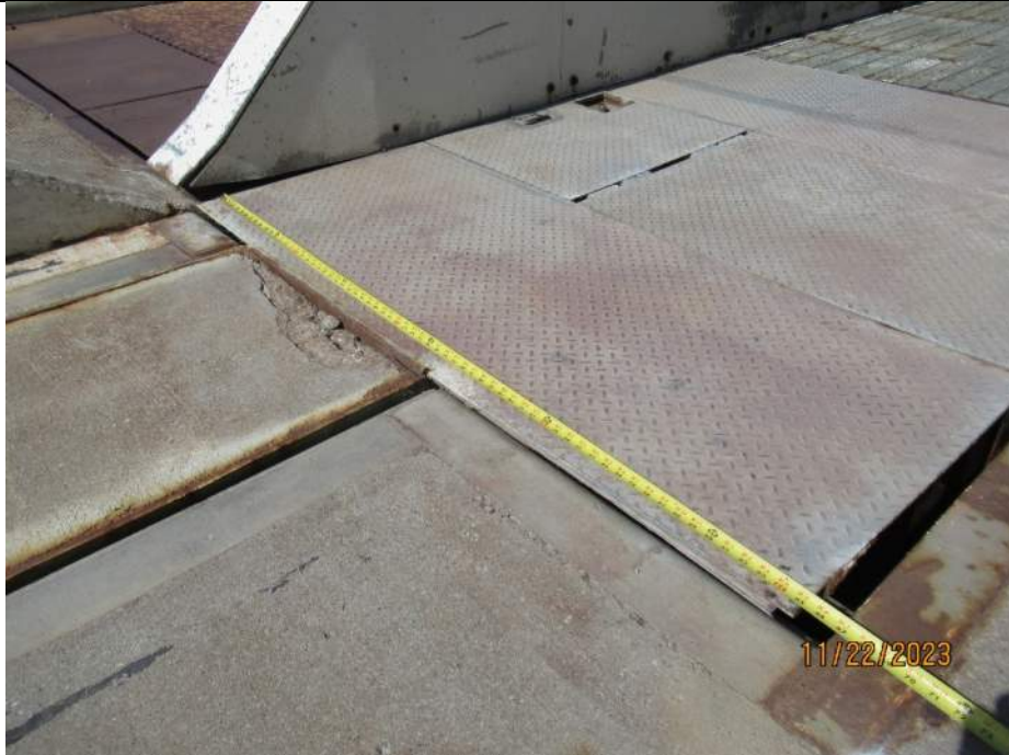
Photo S-143 - [Span 5] -South leaf rear break joint at East sidewalk, diamond plating at longitudinal break is uplifted and presents a minor tripping hazard, Looking Northwest
