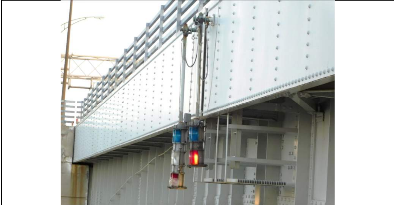
Photo S-323 - [Span 5] -West side navigational lights, north light not functional, south light functional, Looking North
