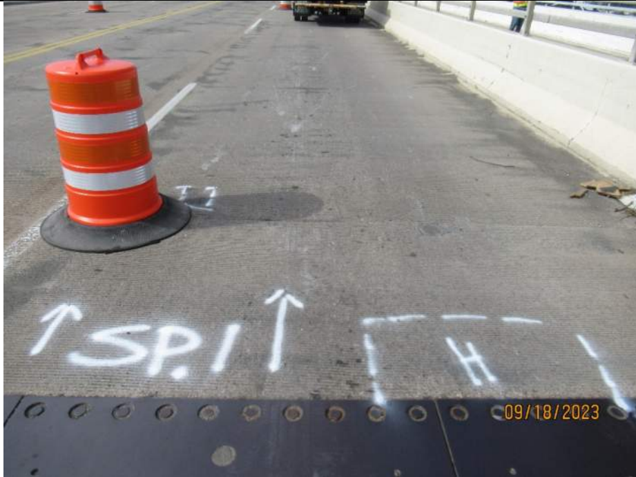
Photo S-35 - [Span 1] -Roadway deck and wearing surface, NB lanes at south end of span, Looking North
