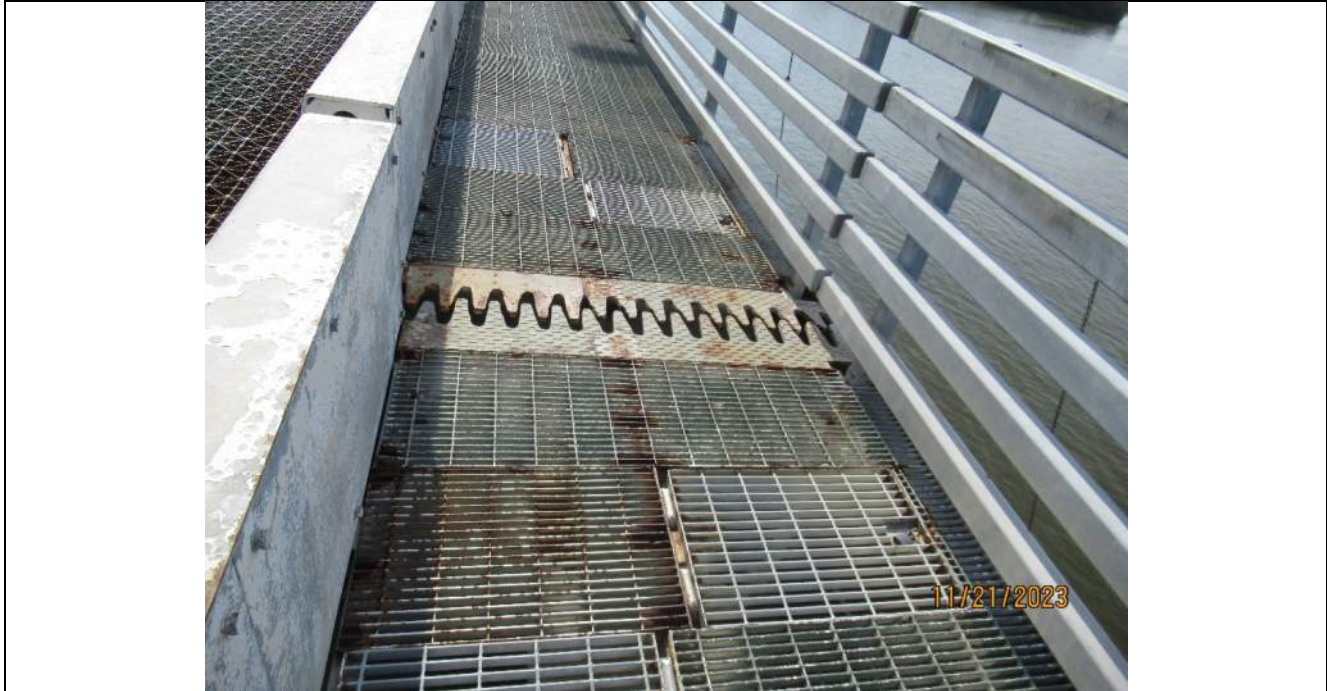
Photo S-141 - [Span 5] -Bascule span center finger joint, detail view at West sidewalk, Looking South
