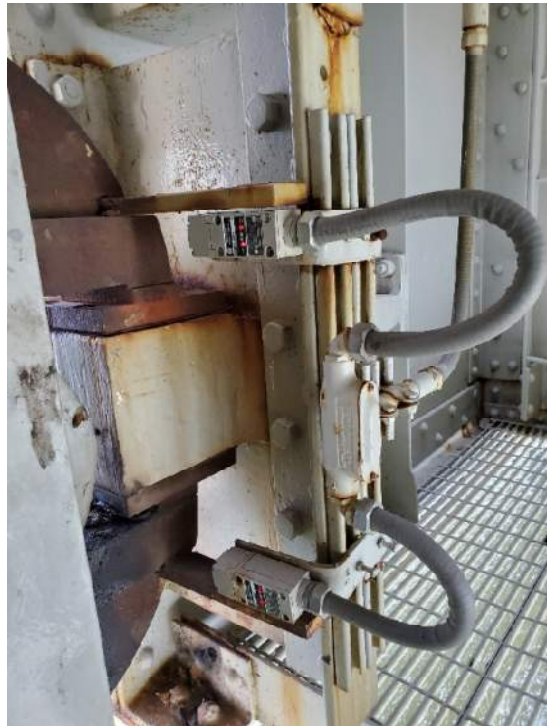
Photo E-20: Span Lock Proximity Switches
