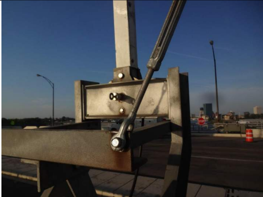
Photo 63 - [NE Traffic Gate] – Note missing jam nut on turnbuckle.
