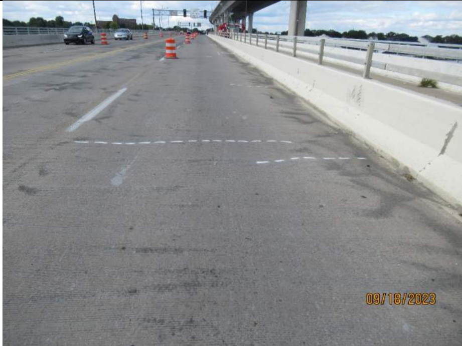
Photo S-39 - [Span 2] -Roadway deck and wearing surface, NB lanes at mid-span, Looking North
