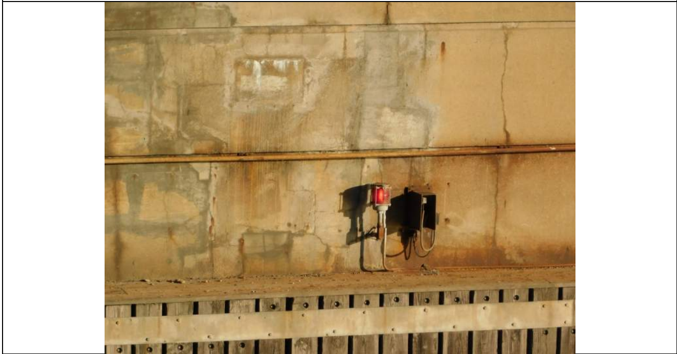
Photo S-324 - [Span 5] -Pier 5 channel side navigational light at center of pier functional, typical for channel lights along both Piers 4 & 5, Looking North
