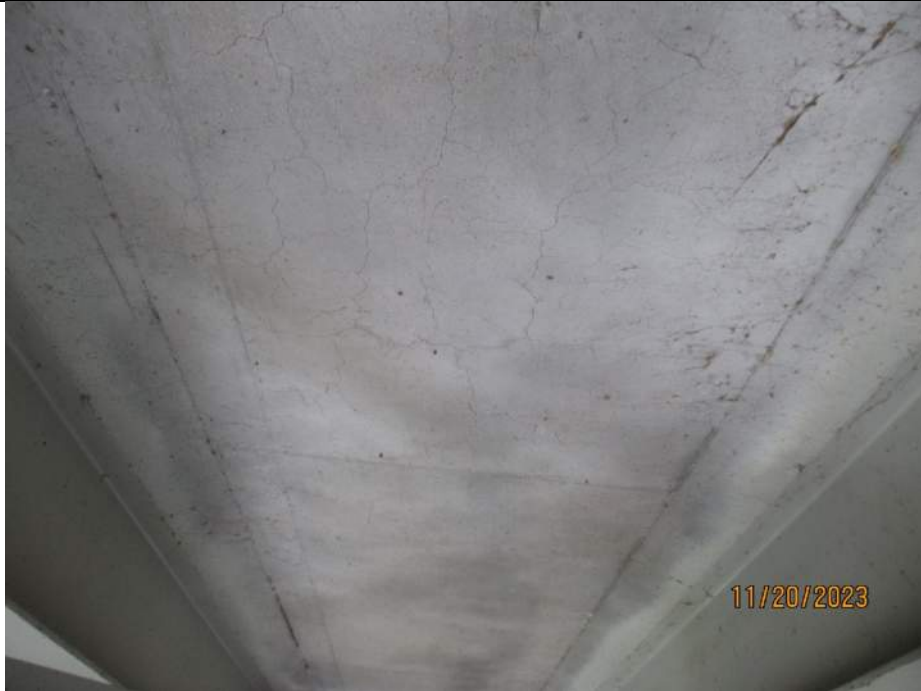
Photo S-161 - [Span 8] -Deck underside, between Stringers 1W-2W and Floorbeams 17S-18S, typical random / map cracking, Looking North
