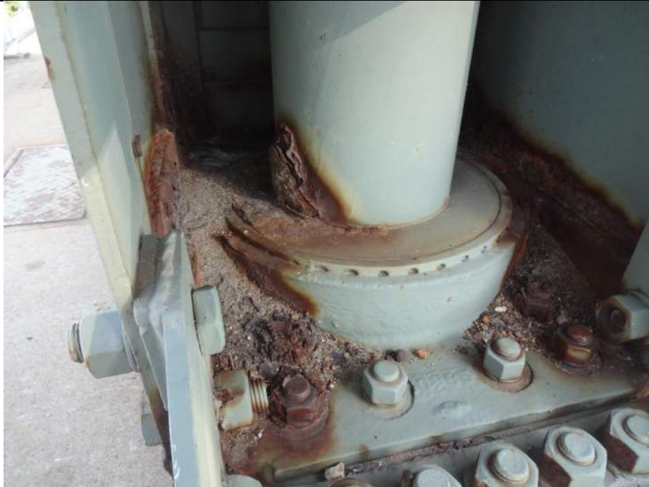
Photo 81 - [NW Swing Gate] – Note severe corrosion on upper bearing fasteners and shaft.
