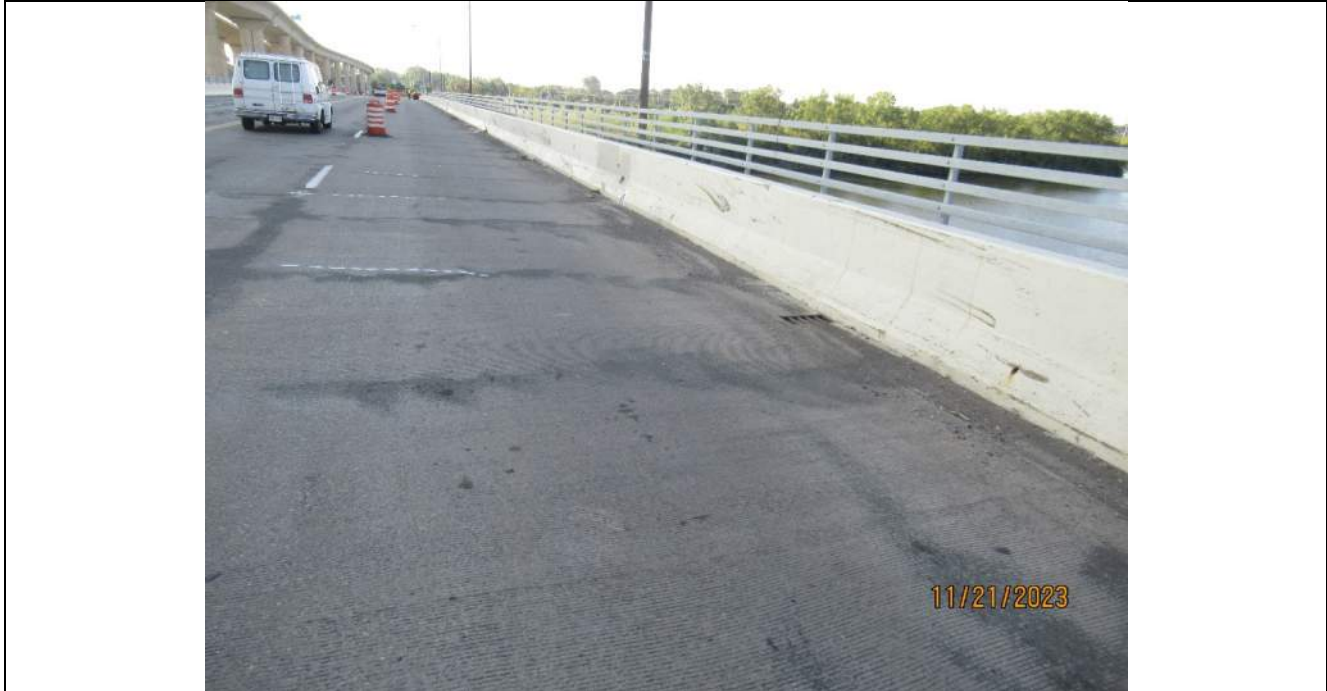
Photo S-49 - [Span 4] -Roadway deck and wearing surface, SB lanes near mid-span, Looking South
