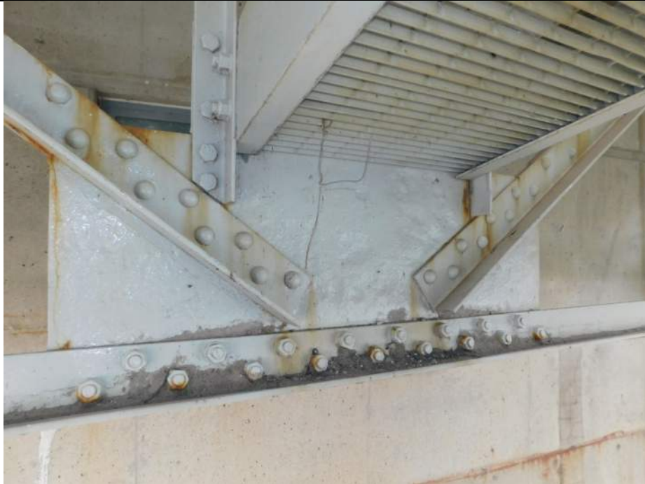
Photo S-245 - [Span 5, North Leaf] -K-bracing below FB7n between G1W-G2W, typical section loss throughout connection plate, Looking North
