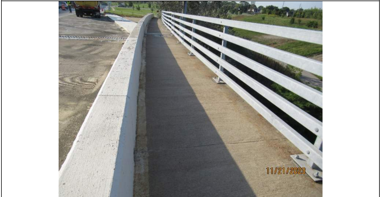
Photo S-102 - [Span 1] -West pedestrian railing and sidewalk, typical good condition, Looking Southwest
