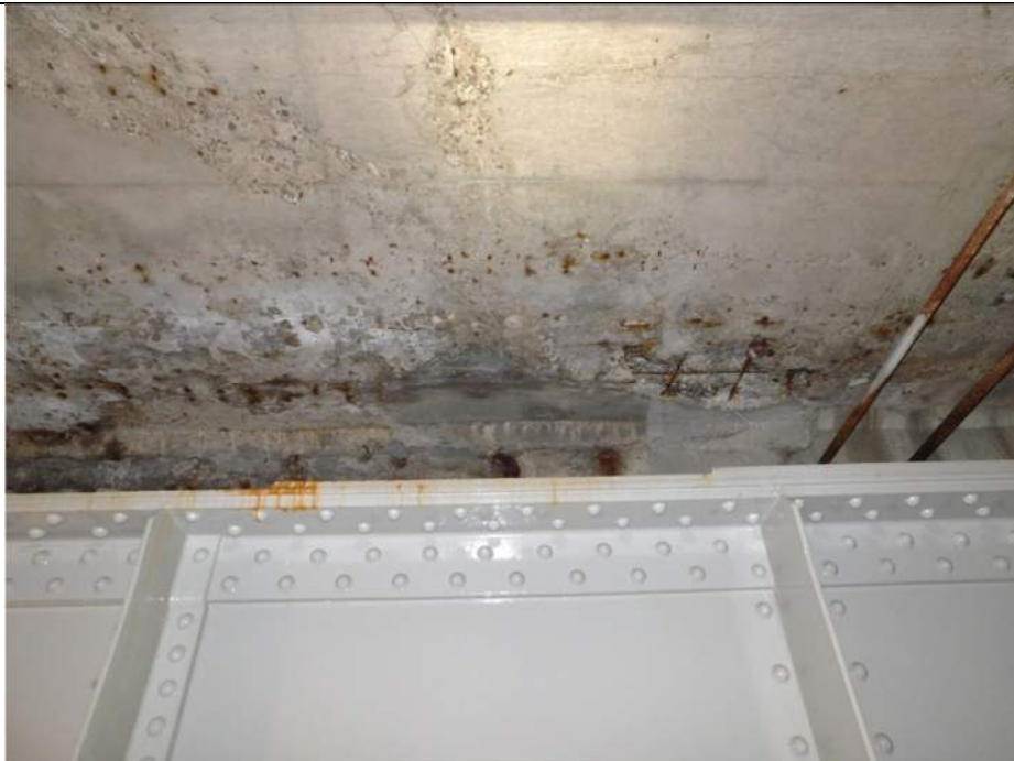
Photo S-346 - [Pier 4 Interior] -Girder 4W at roadway span underside (Level C), view of cracking and small spalls to deck underside above counterweight, Looking West
