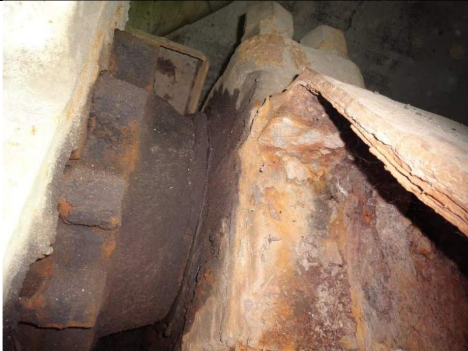
Photo 23 - [NW B1 Bearing] - Severe corrosion is on the inboard side of B1 bearing.
