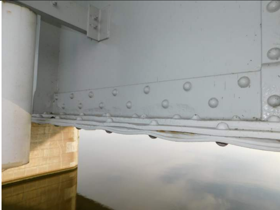
Photo S-177 - [Span 3] -Girder 1W West bottom flange, warping of cover plates due to packing corrosion and isolated section loss to BF angle, Looking Northeast
