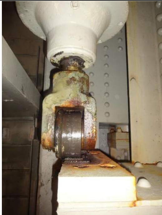
Photo 56 - [NW Seated Buffer] - Seated buffers exhibit transverse misalignment with strike plate as well as some minor surface corrosion.
