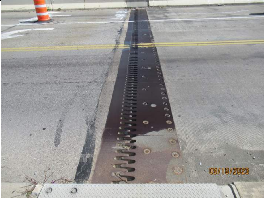
Photo S-131 - [North Abutment] -Abutment reference line finger joint, Span 10 side teeth are 0.25"-0.75" higher than the approach side teeth, primarily in the SB lane, Looking East
