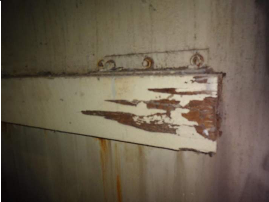
Photo 61 - [North CW Pit] - Wooden counterweight bumpers exhibit isolated fastener corrosion and wood failure.
