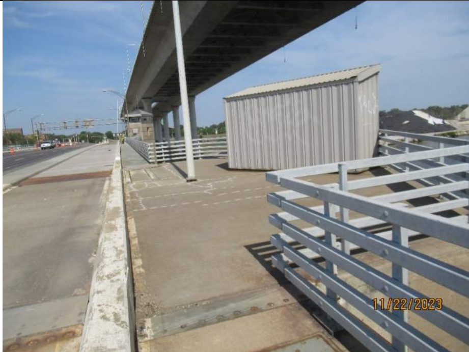
Photo S-107 - [Pier 4 Span] -East sidewalk and railings, good condition general view, Looking North
