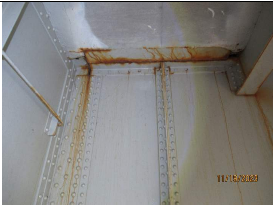
Photo S-194 - [Span 9] -Floorbeam 0S, North face between Stringer 3W and Girder 3W, rust staining and active corrosion across top flange, Looking South
