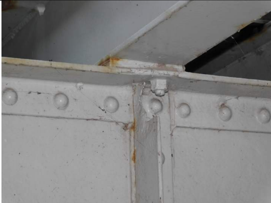
Photo S-217 - [Span 5, South Leaf] -Floorbeam 7s, north side at Stringer 6W, 3" diameter hole in top of web stiffener, Looking South
