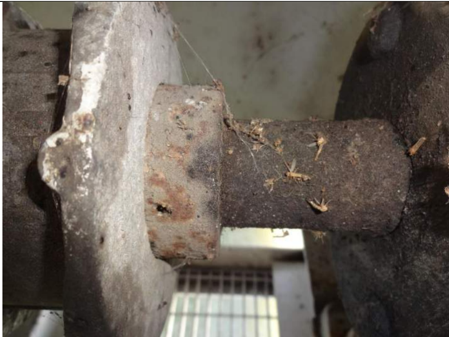
Photo 42 - [Span Locks] - Non-lubricated motor coupling with plugs and gaskets are covered with paint.
