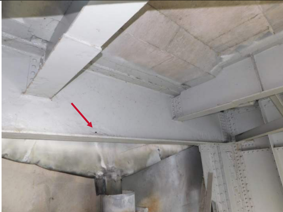
Photo S-189 - [Span 4] -Floorbeam 36S at Pier 4 between Girders 3W and 4W, painted over section loss at lower web with two small holes, Looking Northeast
