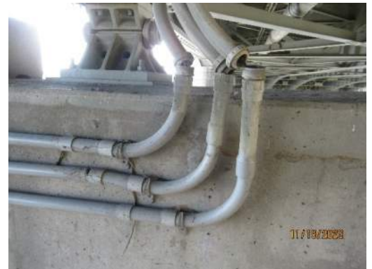
Pier 6 North side, disconnected conduits with rope supports
