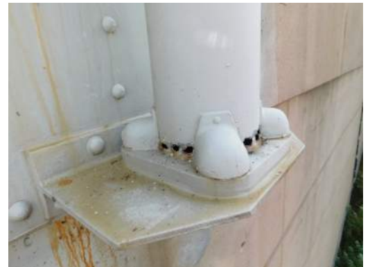
Span 1 West side light pole base with holes
