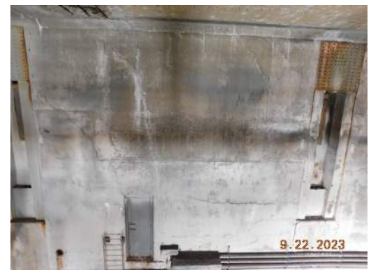
Pier 5 Counterweight Pit Level E upper wall diagonal cracking throughout
