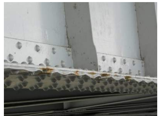
Span 3 Girder 4W east BF pack rust
