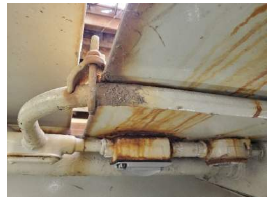
Photo E21: Conduit Near the Southeast Acuator
