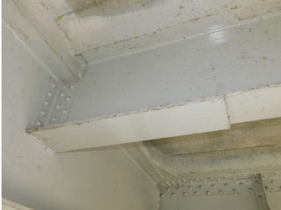
Photo S-201 - [Span 2] -Stringer 6W at connection to Floorbeam 15S, typical welded bottom flange connection plate, stringer, and connections in typical good condition, Looking Northeast
