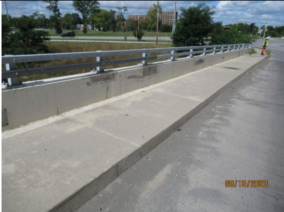
Photo S-120 - [Span 10] -West sidewalk, barrier and railing, minor transverse and vertical cracking, patch repairs to barrier, Looking North
