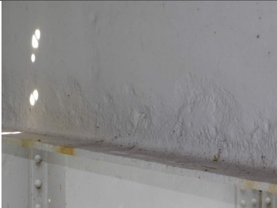
Photo S-219 - [Span 5, South Leaf] -Floorbeam 6s, south face between G3W-G4W, typical section loss throughout lower web and two holes up to 1/4" dia, Looking Northwest
