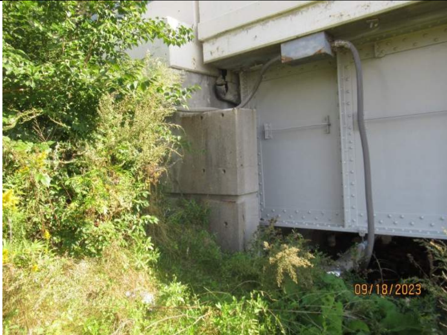
Photo S-281 - [North Abutment] -Abutment backwall and cheek at West wingwall, cracks propagating from corner where walls meet, general view, Looking Northeast
