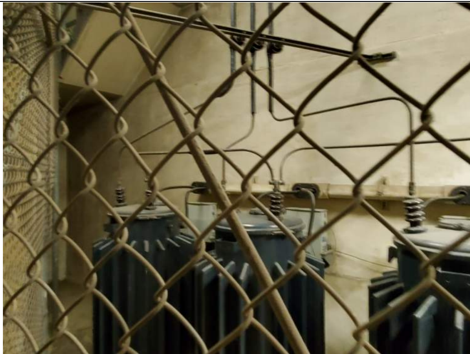
Photo E-02: Medium Voltage Transformers located in a lower level of the Control House
