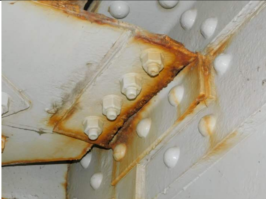
Photo S-241 - [Span 5, South Leaf] -Upper diagonal bracing at FB6s north side to G2W east side, connection angle fully cracked/broken, Looking Southwest
