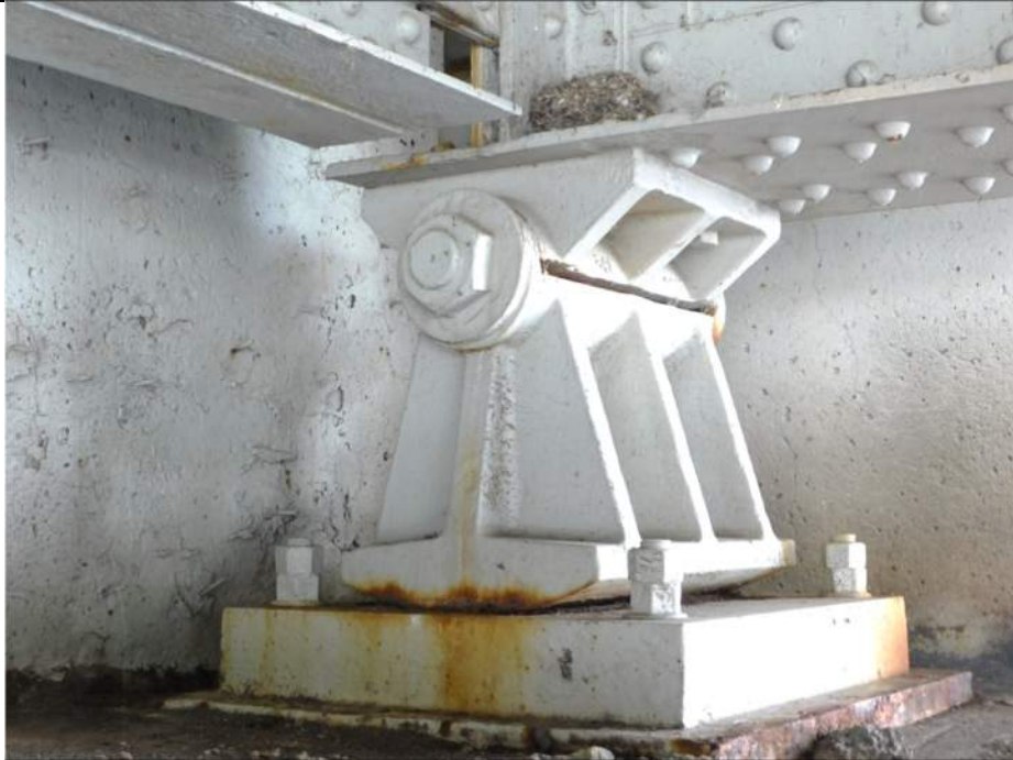
Photo S-259 - [Pier 4] -Bearing 4W at South side of Bascule Pier 4, general view of bearing generally plumb, Looking East
