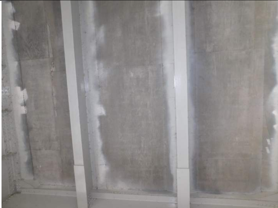
Photo S-153 - [Span 2] -Deck underside, general view between Floorbeams 6S & 7S, Stringers 3S & 4S, Looking South
