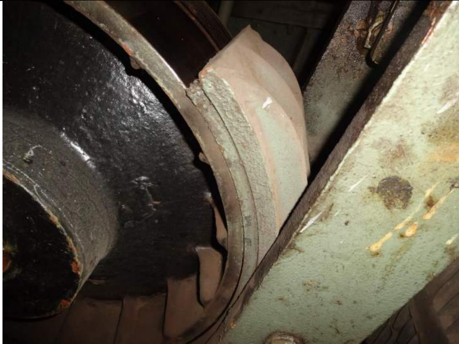
Photo 13 - [SE Motor Brake] - Both the north and south pads stay in contact after release on motor brake, roughly 10% for the north and 25% for the south. South pad is shown.
