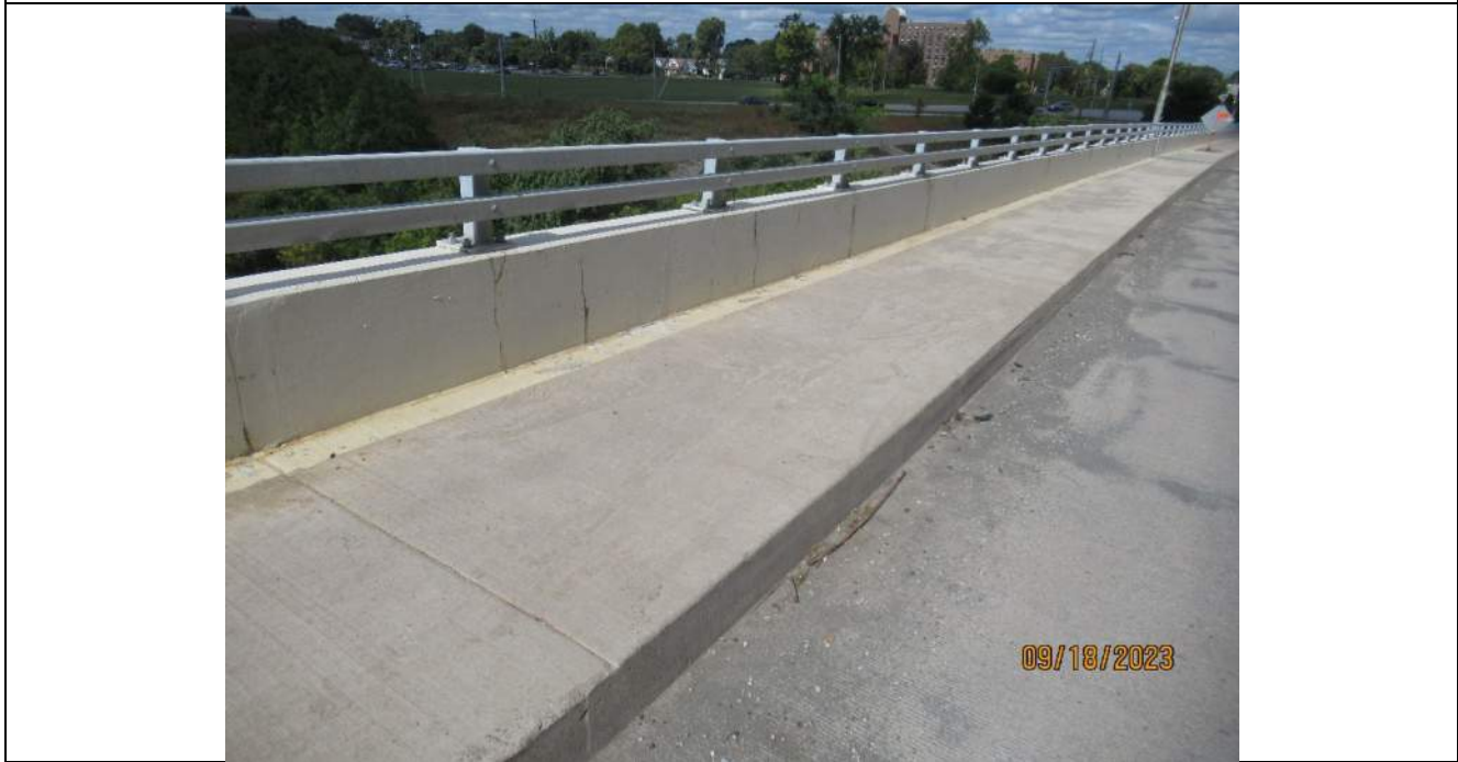
Photo S-118 - [Span 8] -West sidewalk, barrier and railing, minor transverse and vertical cracking, Looking North
