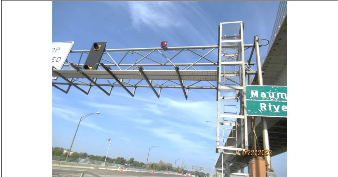
Photo S-326 - [Span 4] -Overhead Sign Gantry, South elevation east half, detail view, components in good condition, Looking North
