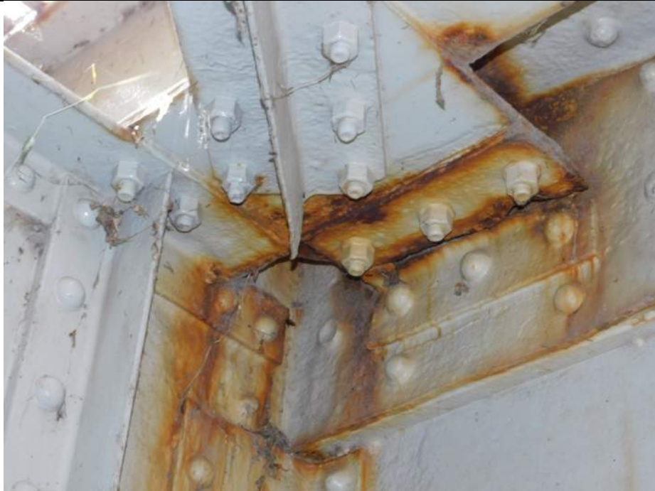
Photo S-237 - [Span 5, South Leaf] -Upper diagonal bracing at FB7s north side to G3W east side, connection angle fully cracked/broken, Looking Southwest
