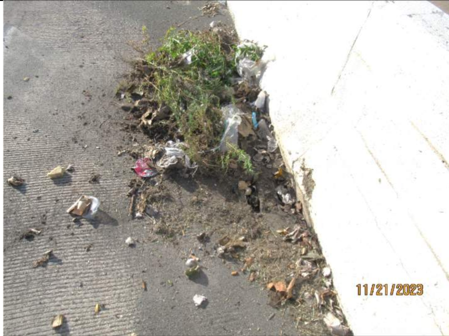
Photo S-147 - [Span 1] -Typical clogged roadway drain next to west barrier, 3rd drain from abutment, Looking South
