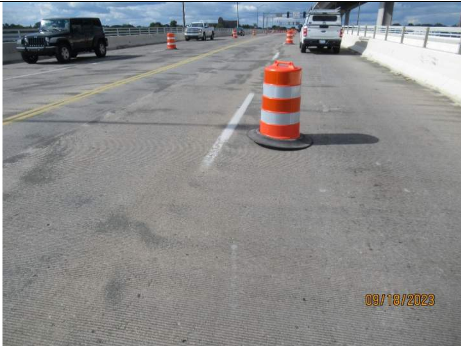
Photo S-36 - [Span 1] -Roadway deck and wearing surface, NB lanes at mid-span, Looking North
