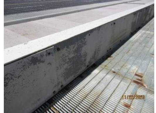
Span 5 south leaf east trail to sidewalk barrier, missing bolts at vertical plate
