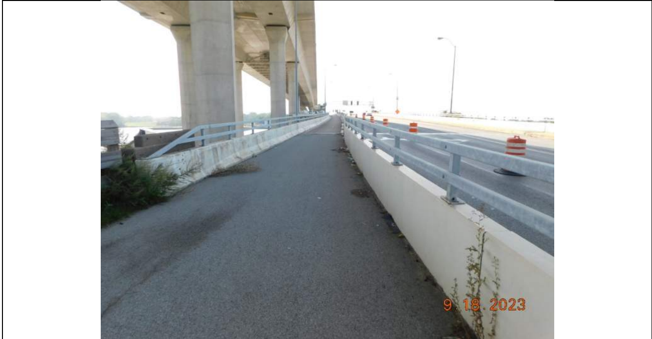
Photo S-15 - [North Approach] -East sidewalk / trail approach pavement, general view, Looking South
