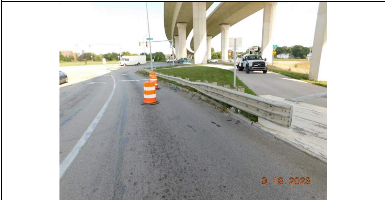
Photo S-28 - [North Approach] -Northeast guard railing transition and barrier, minor impact damage, Looking Northeast
