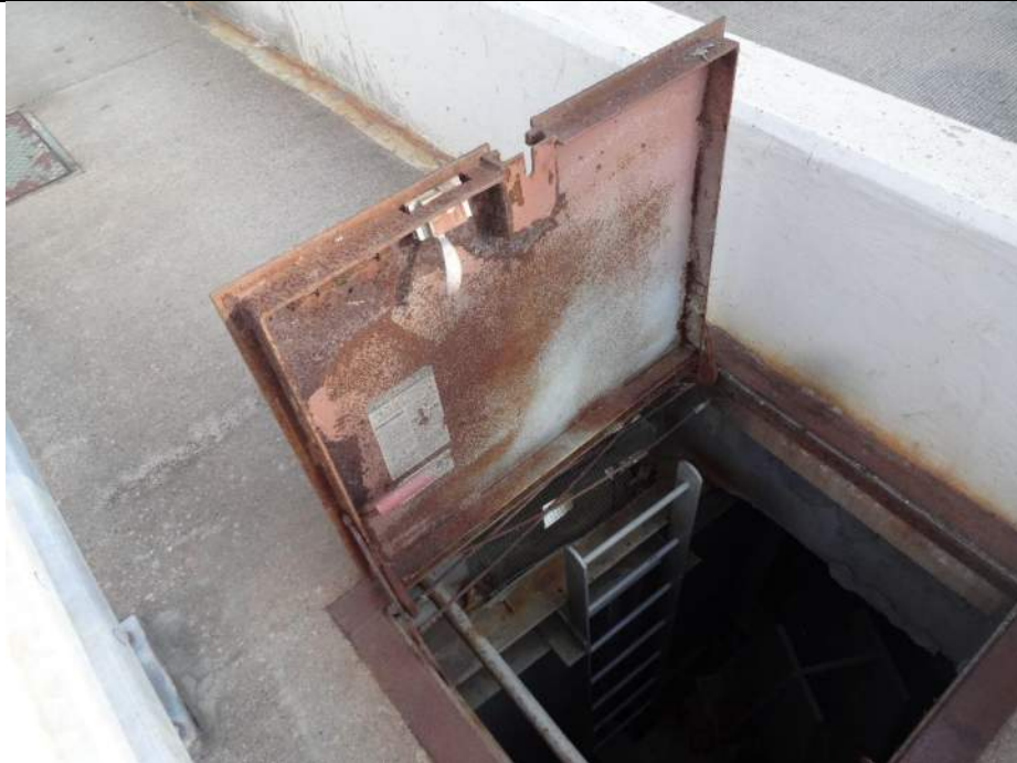
Photo 75 - [SE Swing Gate] - Heavy corrosion is present on access doors and hinges to access swing gate machinery.
