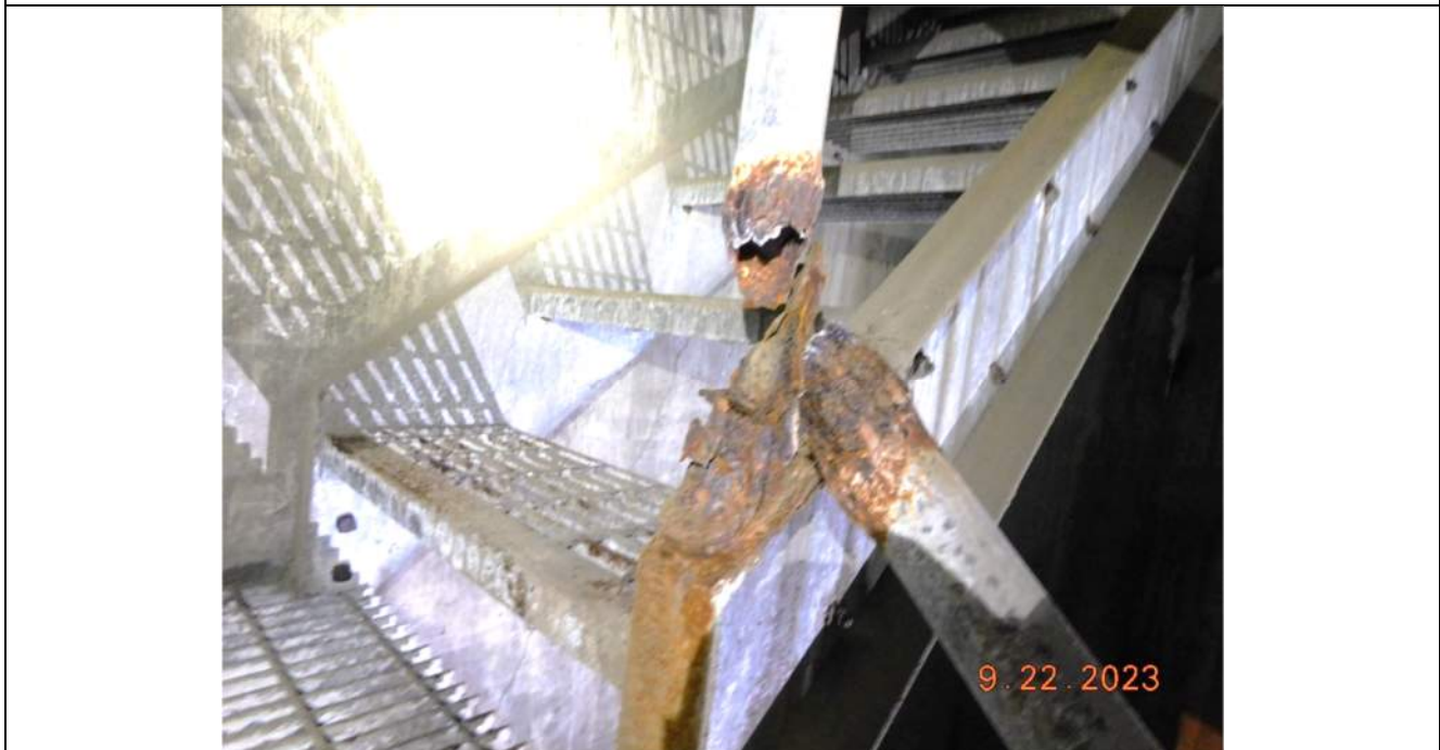
Photo S-368 - [Pier 5 Interior] -Level F, mid-level of stairs in East exterior room, 100% section loss to post and railing, Looking South
