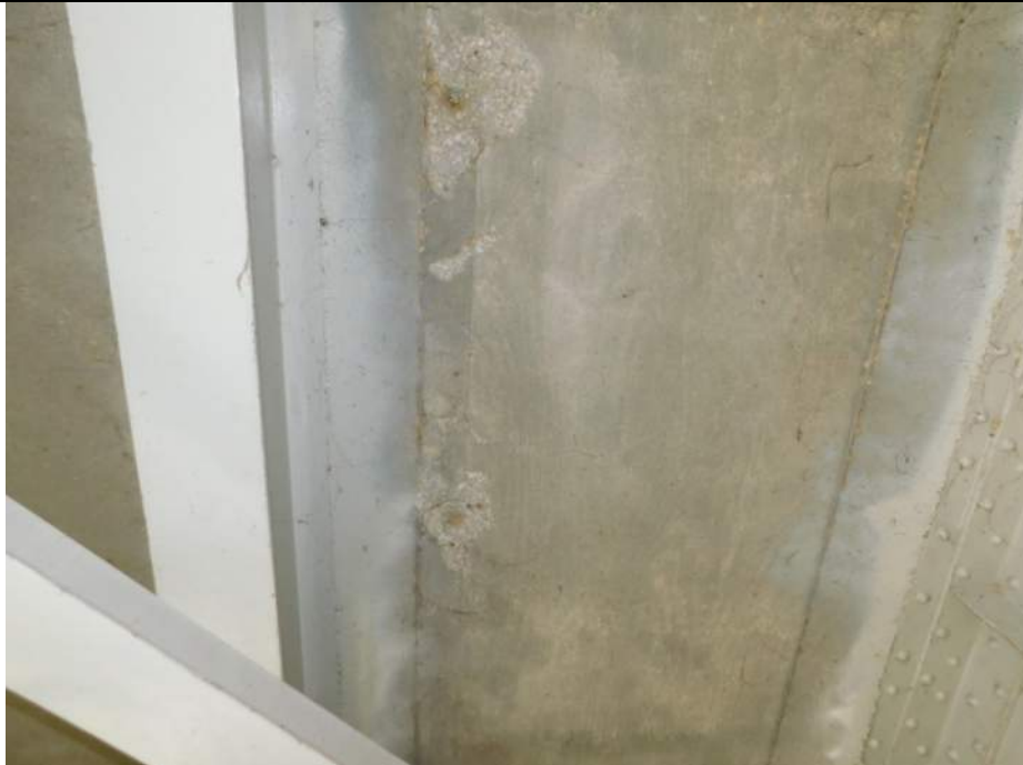
Photo S-156 - [Span 2] -Deck underside, between Floorbeam 9S-10S and Stringers 5W-6W, minor pop-out spalls in deck (below trail-roadway barrier), Looking South
