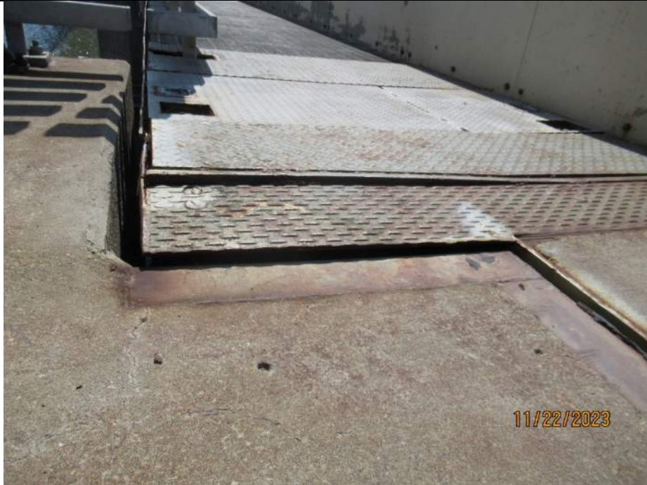
Photo S-111 - [Span 5] -North leaf east sidewalk at north end, vertical misalignment along longitudinal and transverse breaks presents minor tripping hazard, Looking South
