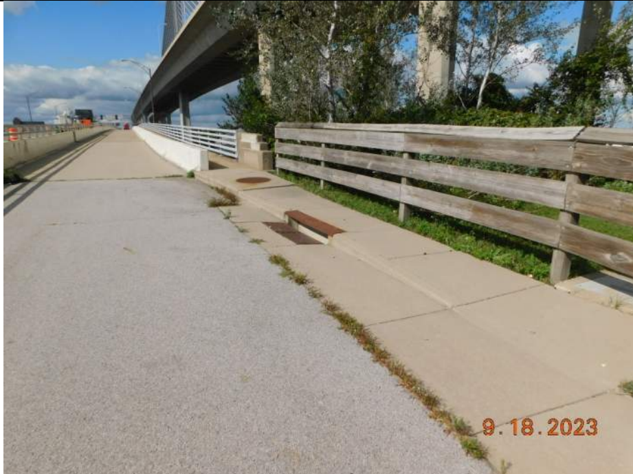
Photo S-33 - [South Approach] -Southeast drain inlet at east side sidewalk / trail, general view, Looking Northeast
