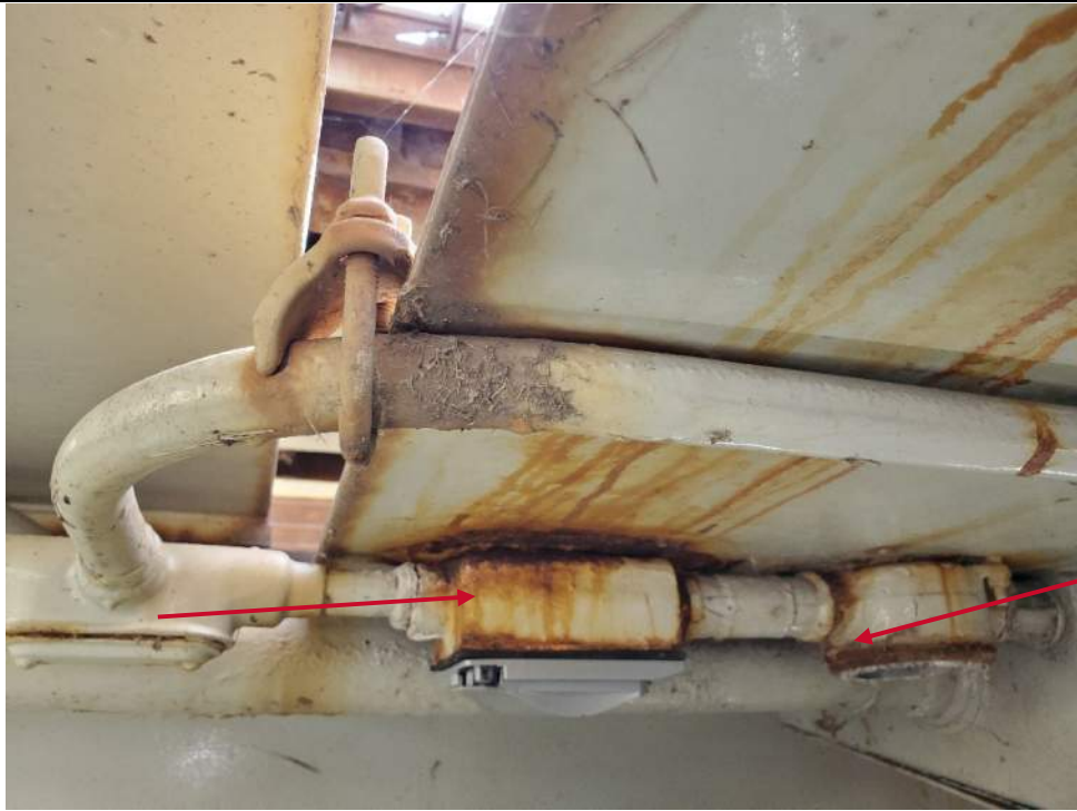
Photo E-21: Conduit near the Southeast Traffic Gate Actuator. Note the corrosion.
