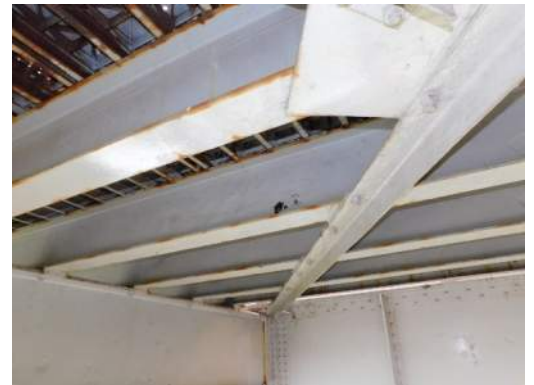
Span 5 South leaf, Stringer 26W web hole
