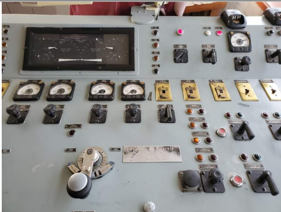
Photo E-16: Control Console
