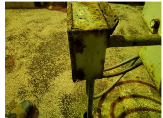
Photo E12: Motor Brake Junction Box
