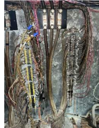
Photo E22: South Pier Submarine Cable Termination Cabinet
