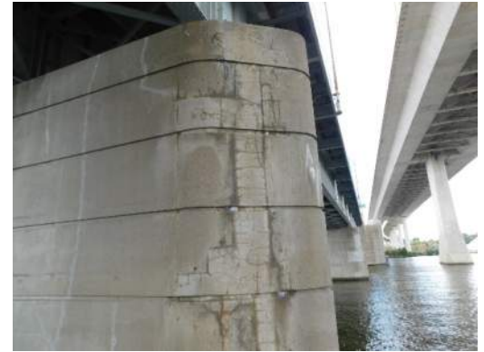
Pier 3, South side at East end, cracking in patched areas
