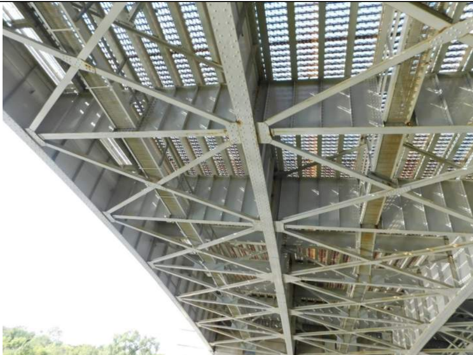
Photo S-166 - [Span 5] -Span framing and underside general view, North leaf, Girders 1W-3W, Looking North
