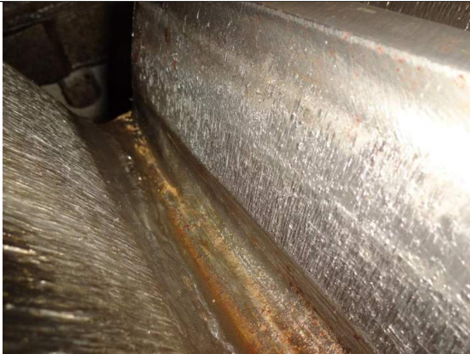
Photo 26 - [South Machinery Room] – Note severe scoring across all open gear faces on both sides.
