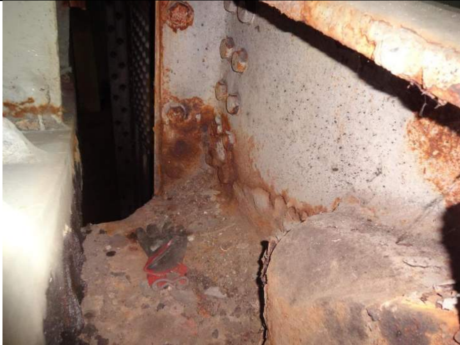
Photo 25 - [NE B1 Bearing] - Moderate surface corrosion is present on fasteners and inboard side of B1 bearing anchorage.
