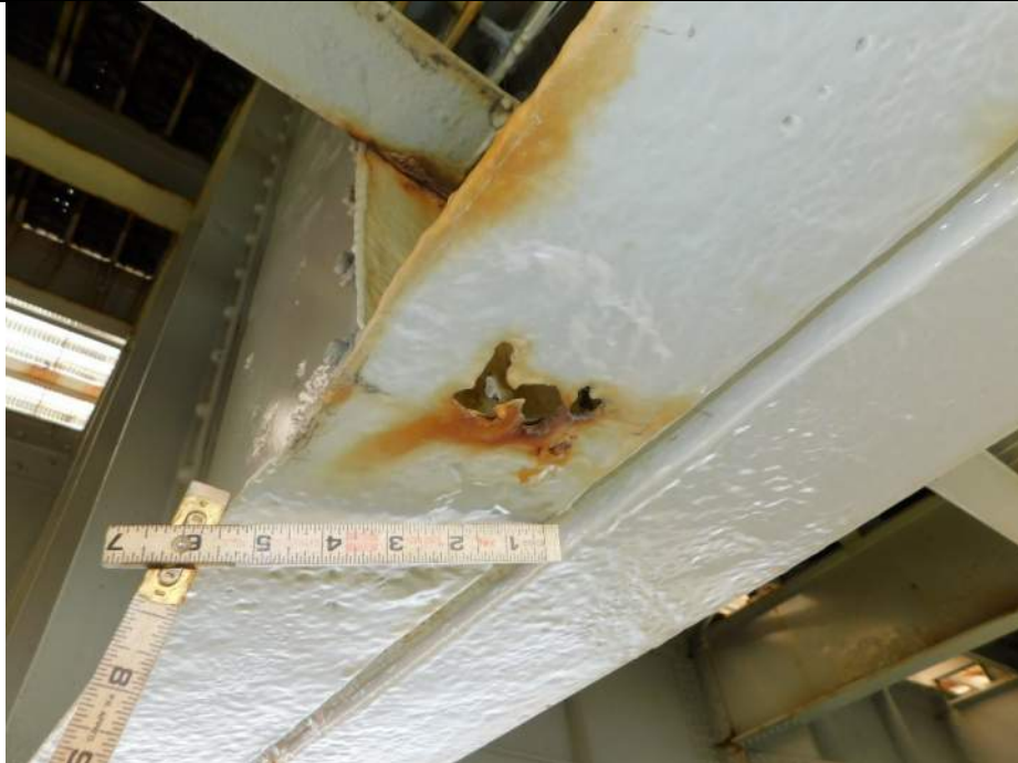
Photo S-223 - [Span 5, South Leaf] -Floorbeam 3s between G3W-G4W, north BF with 2"x1" hole below catwalk, Looking Southeast
