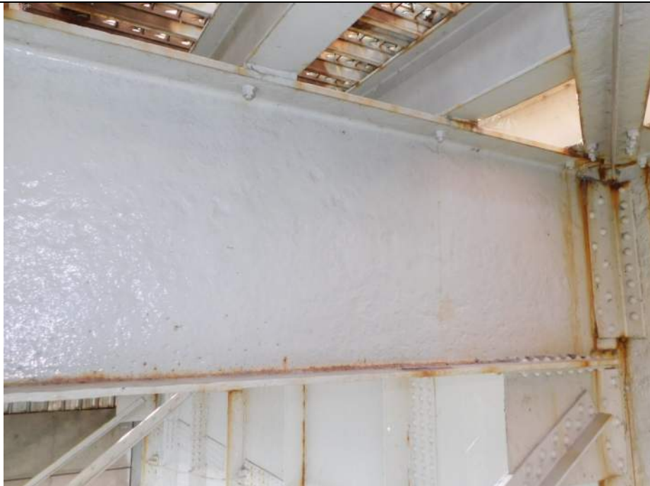
Photo S-220 - [Span 5, South Leaf] -Floorbeam 5s north face at G3W, detail view of typical web section loss with spots up to 1/4" deep, Looking Southwest
