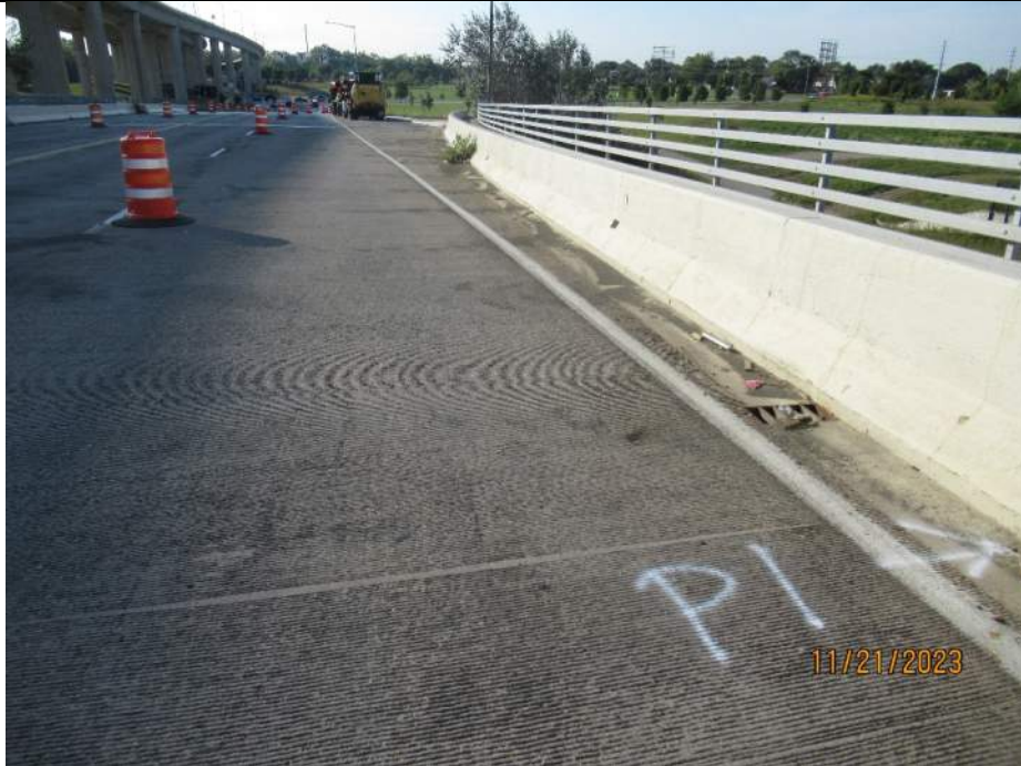
Photo S-83 - [Span 1] -West roadway barrier, typical vertical cracking, Looking Southwest
