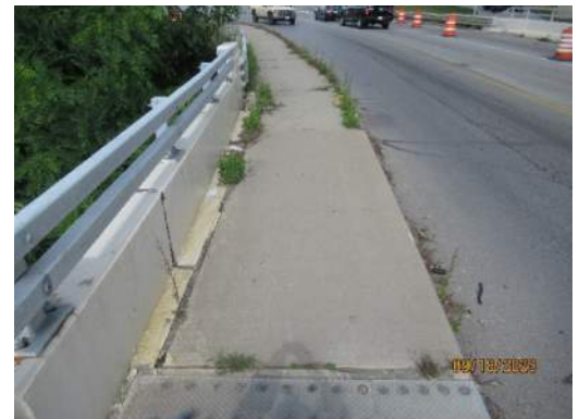
Northwest sidewalk vegetation growth
