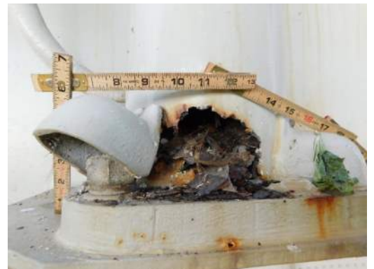
Span 1 East side light pole base with holes
