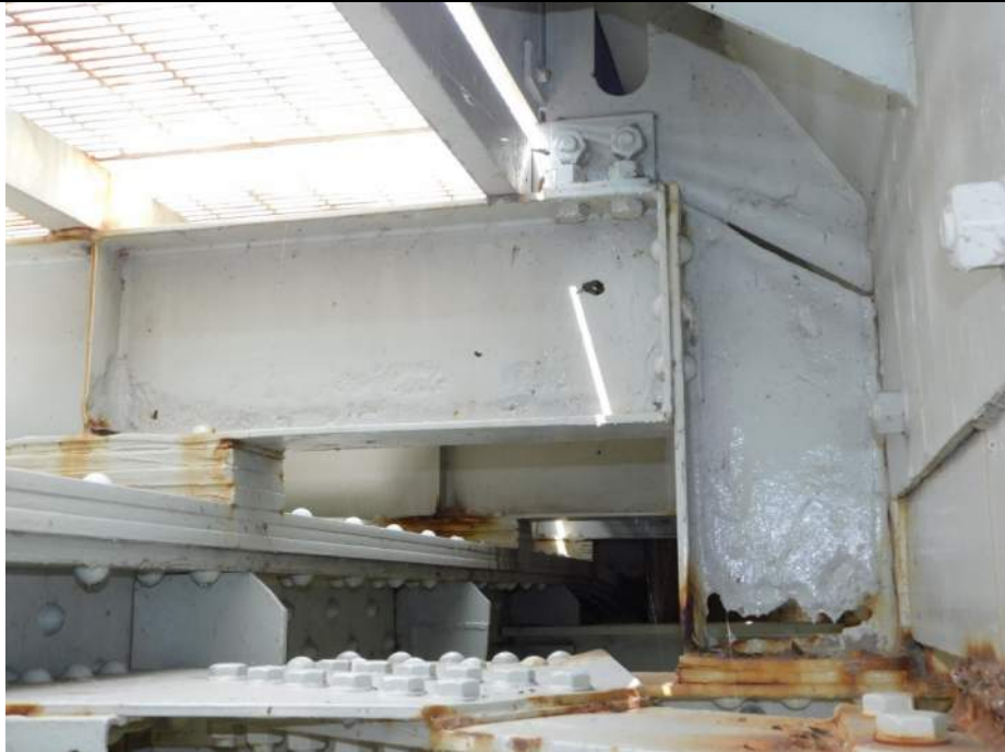
Photo S-250 - [Span 5, North Leaf] -West sidewalk support beam and post at FB7n, holes in beam web and base of post, Looking North
