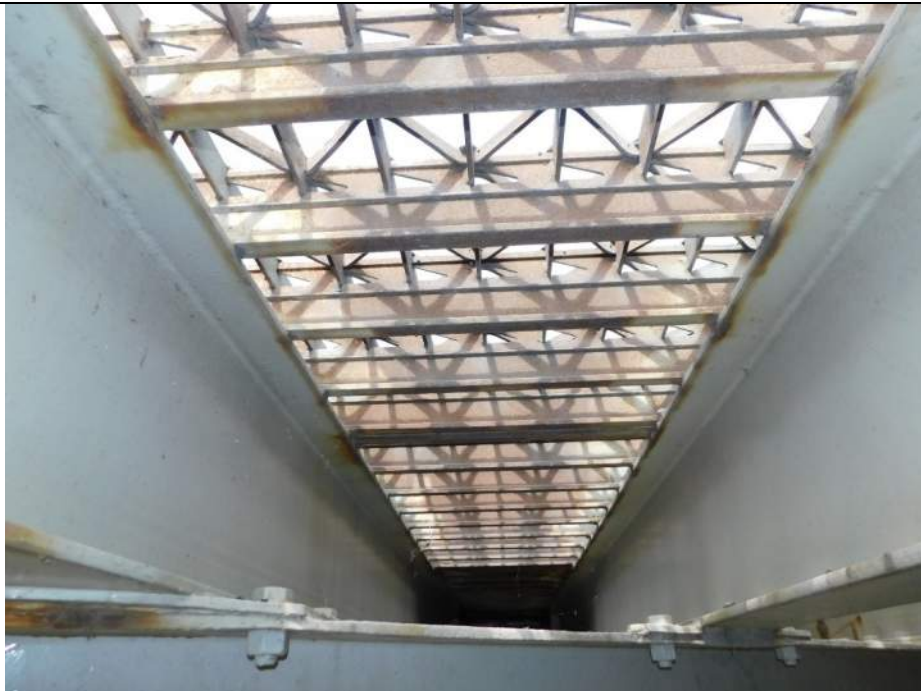
Photo S-234 - [Span 5, North Leaf] -Stringers 7W-8W and grid deck lower main bars, between FB6n-FB7n, general view of typical good condition, Looking North
