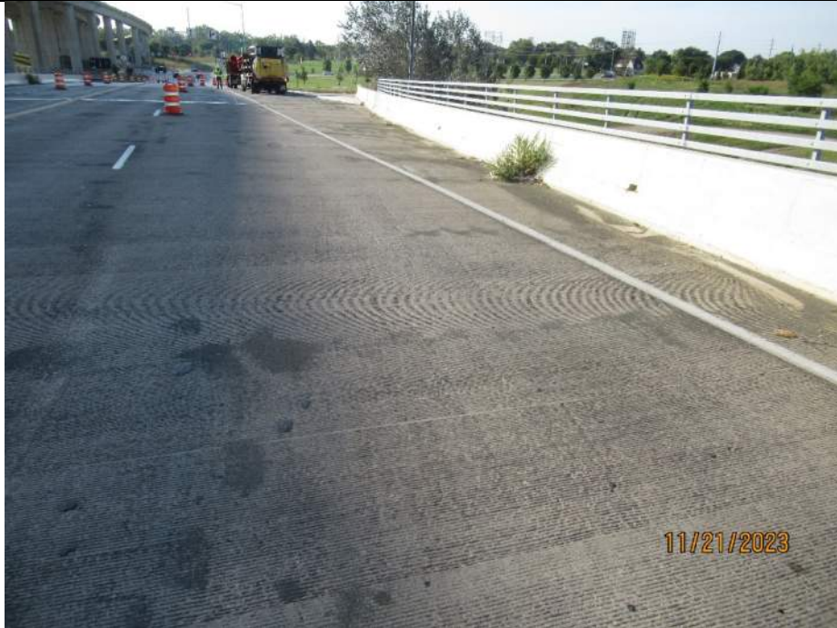
Photo S-37 - [Span 1] -Roadway deck and wearing surface, SB lanes near north end of span, Looking South
