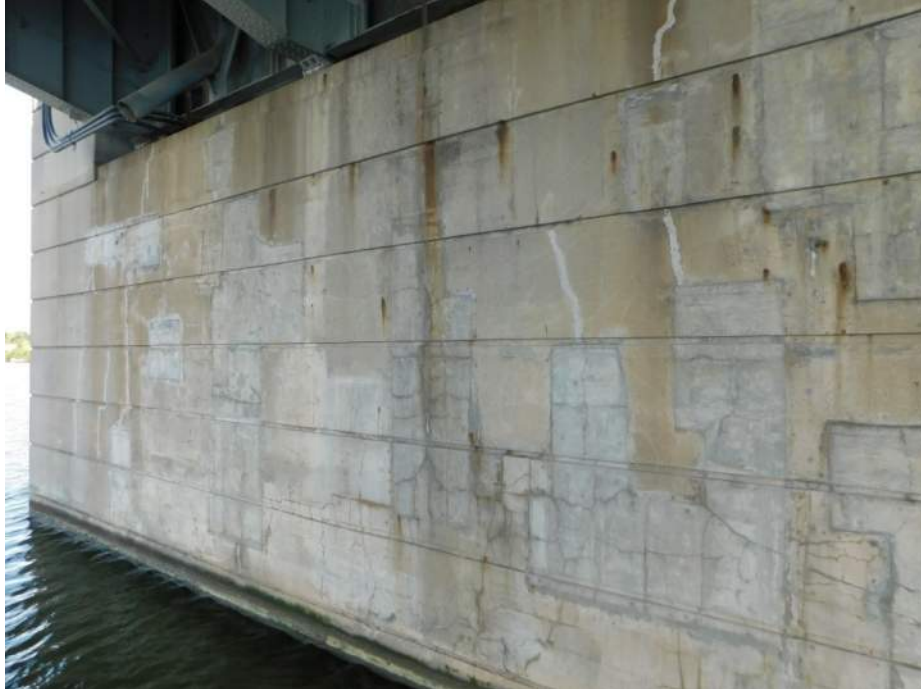
Photo S-295 - [Pier 4] -Pier South face, detail view of widespread patch and crack repairs, cracking in and around repair areas, Looking Northwest
