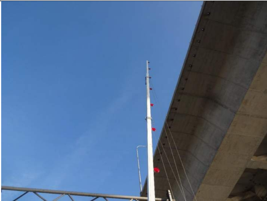
Photo 62 - [NE Traffic Gate] - Vertical traffic gates have loose guy wires.
