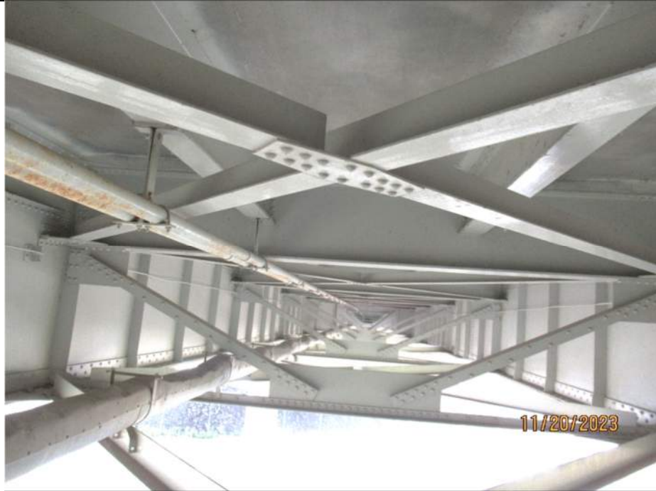
Photo S-209 - [Span 8] -General view of diagonal and transverse bracing between Girders 3W and 4W from FB19S, Looking South
