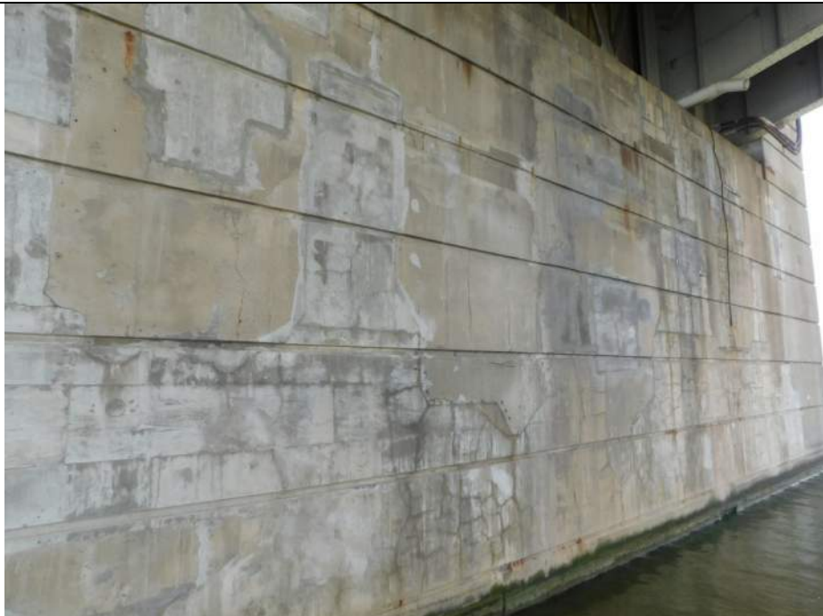
Photo S-304 - [Pier 5] -Pier North face, detail view of widespread patch repairs with scattered cracking, Looking Southwest
