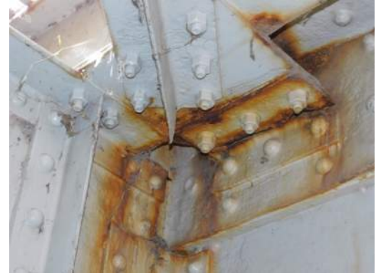
Span 5 South leaf, upper diagonal at FB7s north side to G3W east side
