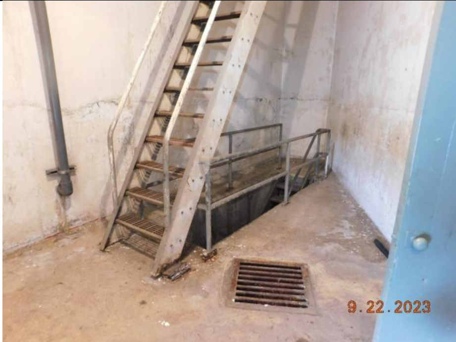
Photo S-369 - [Pier 5 Interior] -Level E, East exterior room, packing corrosion at railing and stairs connections to floor, Looking South
