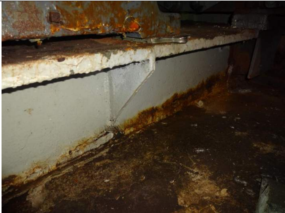
Photo 4 - [North Machinery Room] – Note surface corrosion on base of motor support and use of finger shims.
