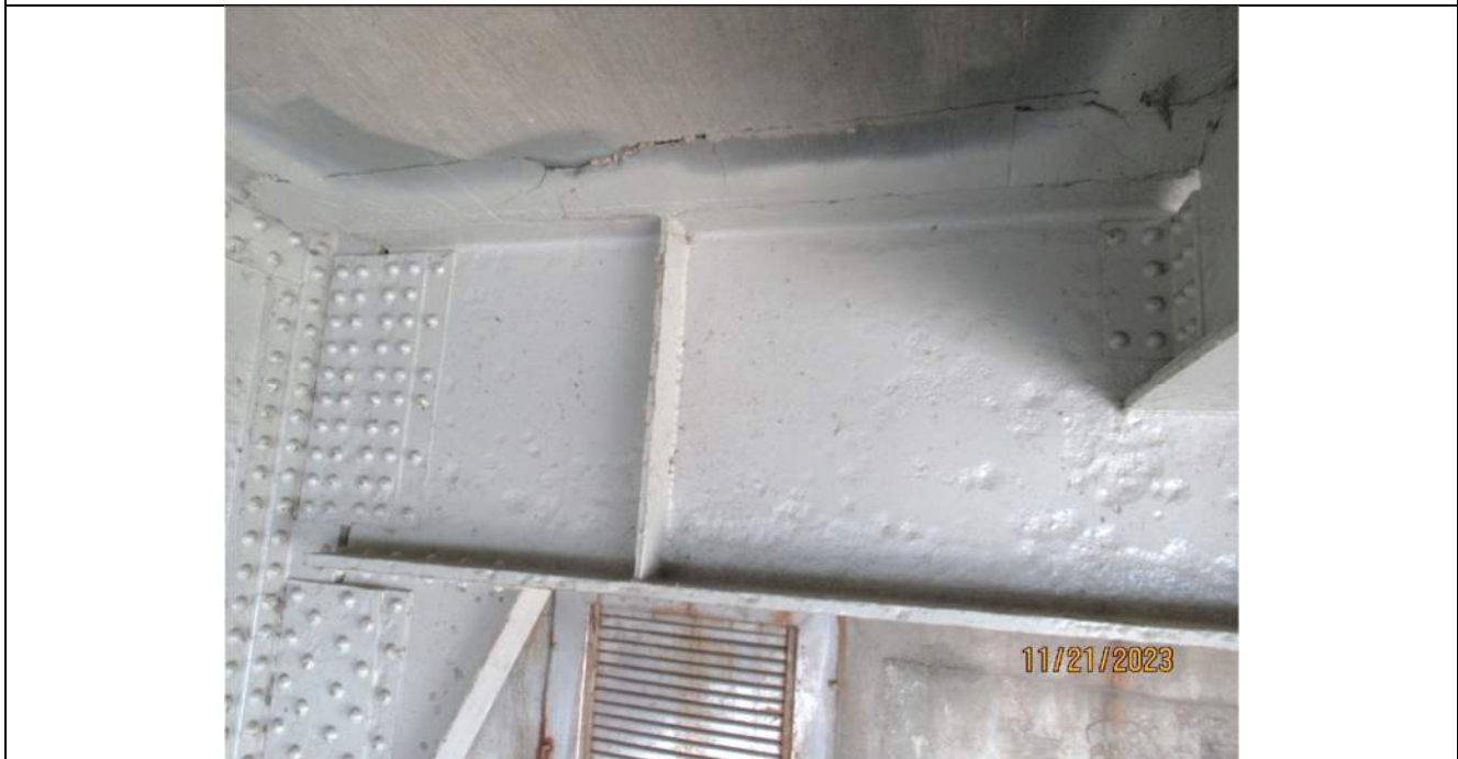
Photo S-186 - [Span 1] -Floorbeam 0S at the South Abutment widespread painted over deep section loss to the web and flanges, area next to Girder 3W, Looking South
