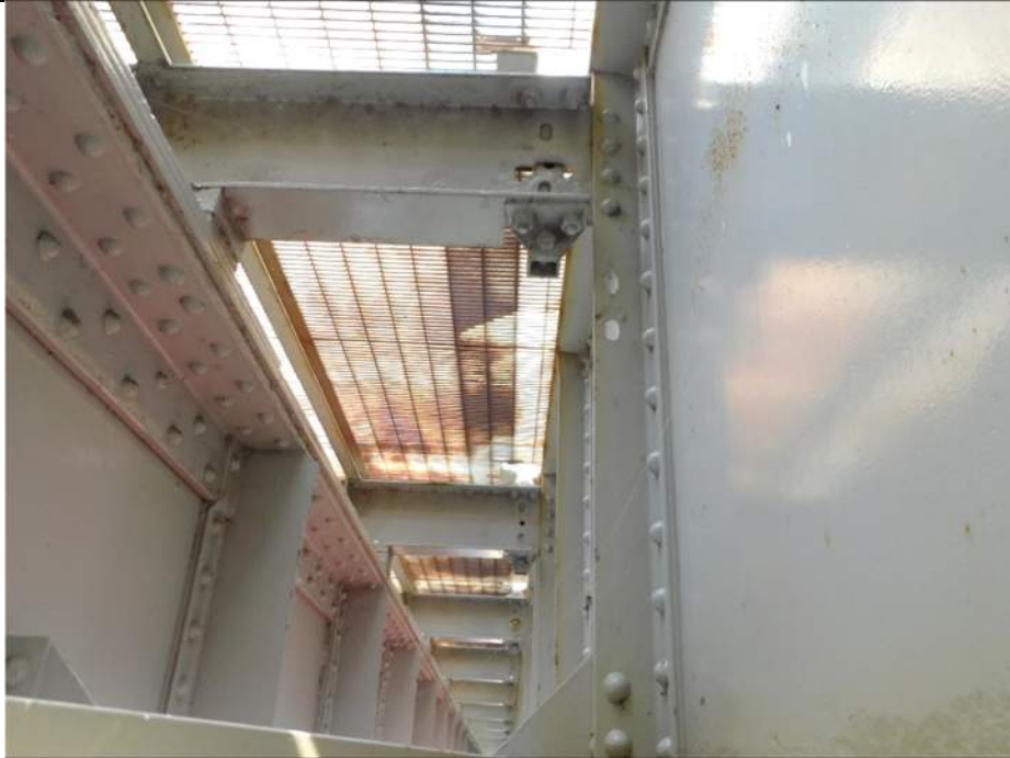
Photo S-249 - [Span 5, South Leaf] -East sidewalk and railing support beams with scattered corrosion holes in webs between FB7s-FB5s, Looking North
