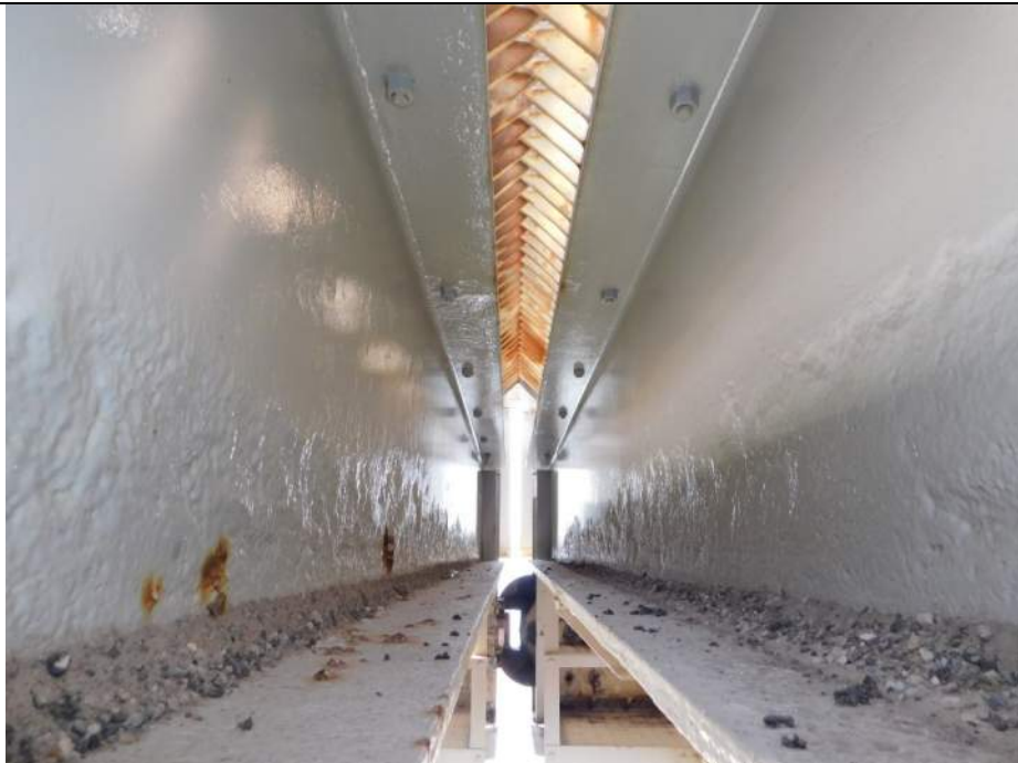
Photo S-226 - [Span 5, North Leaf] -Floorbeams 0n+0s at center break joint between G1W-G2W, typical section loss across lower webs and minor debris accumulation, Looking West
