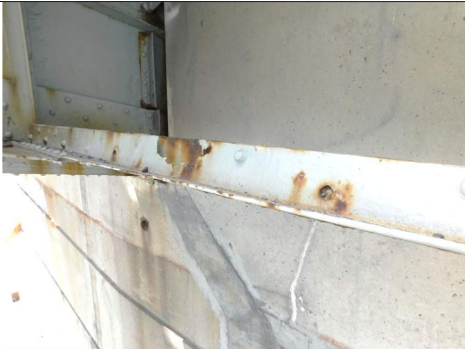
Photo S-246 - [Span 5, North Leaf] -K-bracing below FB7n between G2W-G3W, typical section loss and packing corrosion throughout members, including large hole in angle, Looking West
