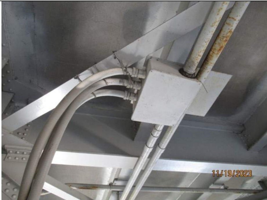
Photo S-336 - [Pier 6] -Three disconnected conduits at north face of pier are supported by rope at upper and lower diagonals, Looking South
