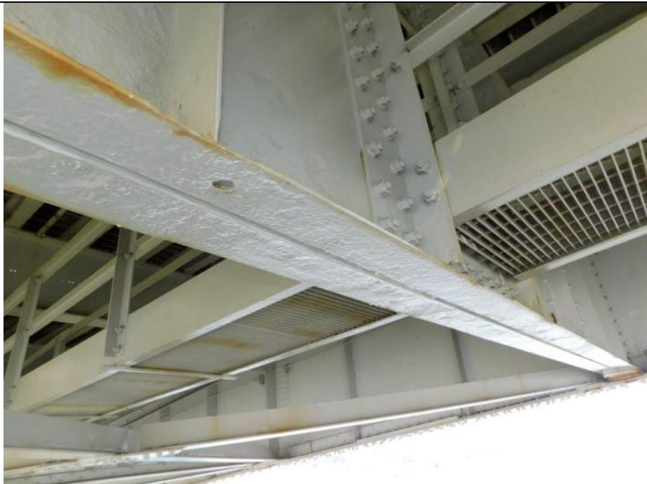
Photo S-230 - [Span 5, North Leaf] -Floorbeam 3n between G3W-G4W, south BF with 1" dia hole and holes in stiffener bases, Looking Northeast
