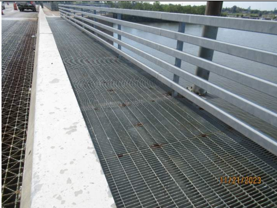
Photo S-108 - [Span 5] -South leaf west sidewalk and railing, typical good condition with spots of corrosion, Looking South
