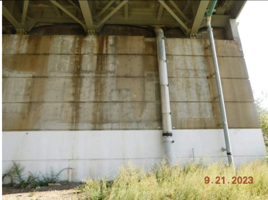
Photo S-273 - [South Abutment] -Abutment stem and back wall view between Girders 1W-3W, Looking South
