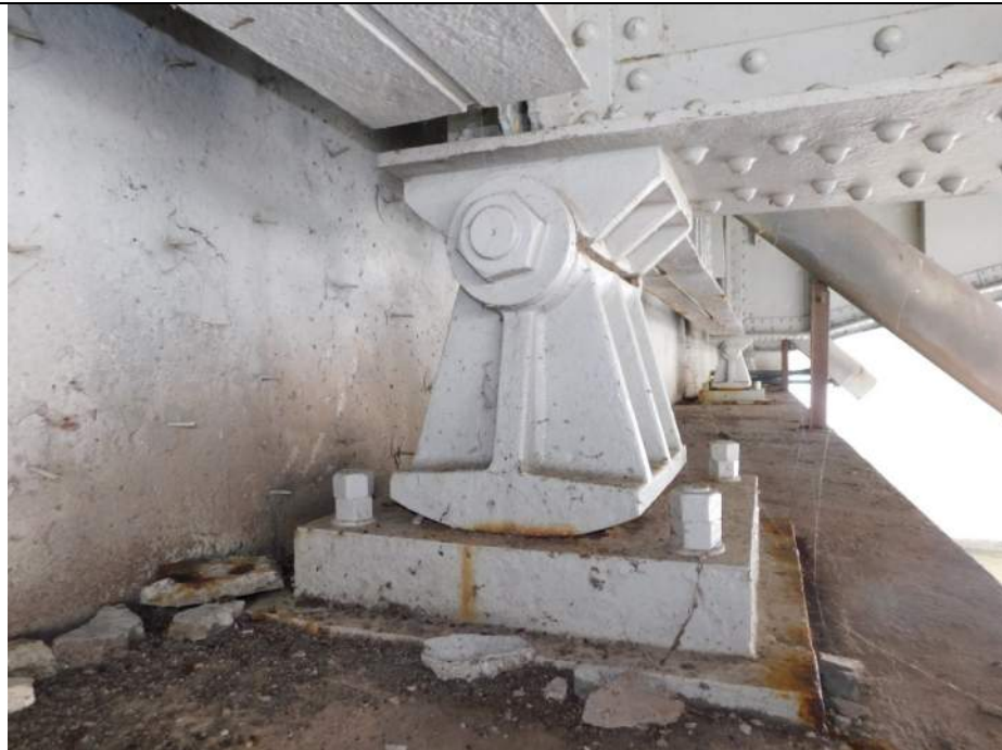
Photo S-258 - [Pier 4] -Bearing 2W at South side of Bascule Pier 4, general view of bearing generally plumb, Looking East
