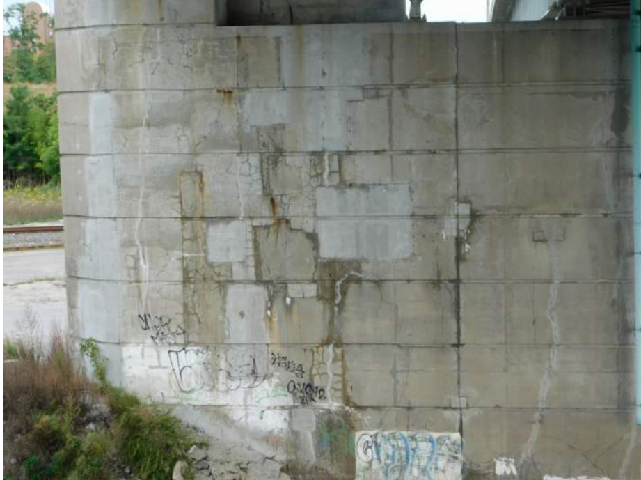
Photo S-307 - [Pier 6] -Pier South face, detail view of west side patch and crack repairs throughout with scattered cracking, Looking North
