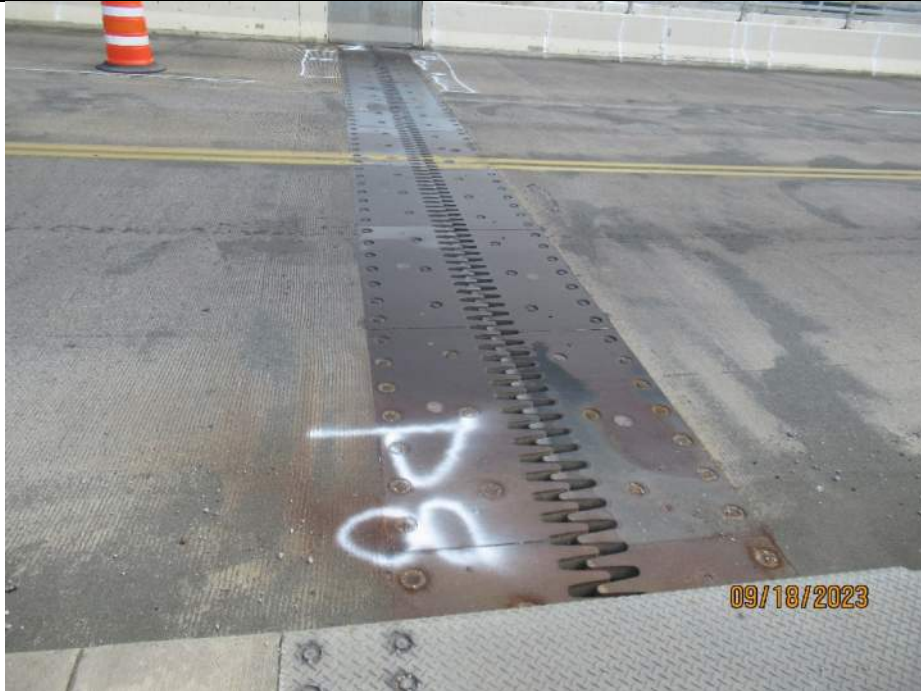
Photo S-145 - [Pier 8] -Expansion finger joint general view across roadway lanes, Looking East
