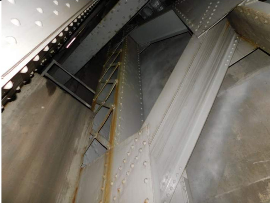
Photo S-353 - [Pier 4 Interior] -Tower 4W East leg at mid-height, North column with scattered painted over section loss throughout, Looking Northeast
