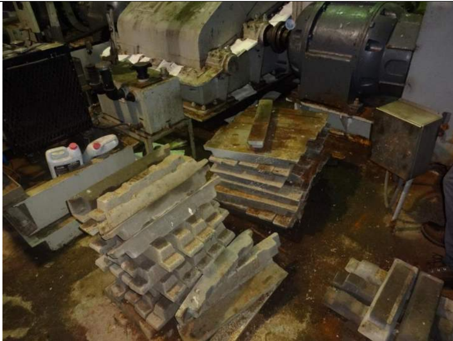
Photo 82 - [North Machinery Room] - Counterweight stacks are present throughout machinery rooms.
