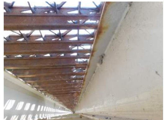
Grid deck main bar corrosion holes
