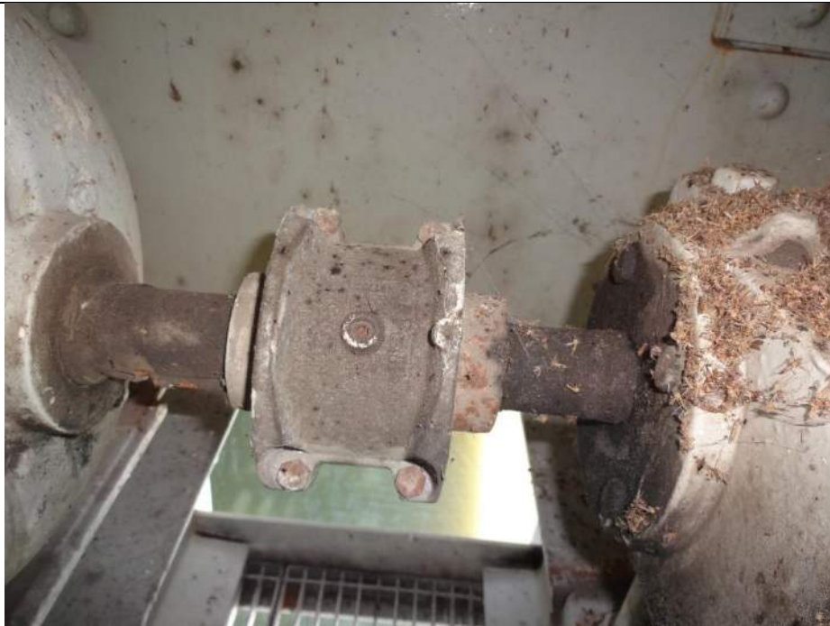
Photo 40 - [Span Lock Motor] – Note heavy corrosion on motor shafts and keys.
