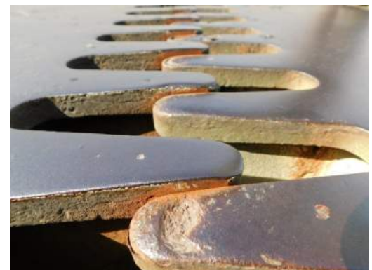
Span 5 center break joint fingers in contact
