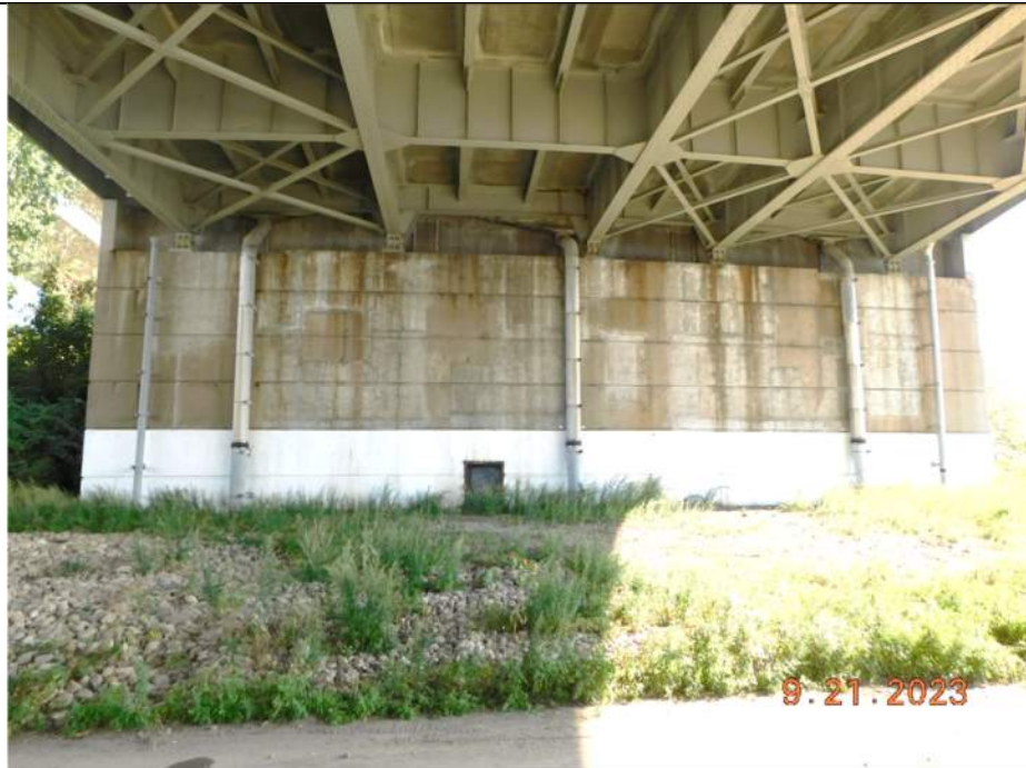
Photo S-272 - [South Abutment] -Abutment stem and back wall general view, Looking South
