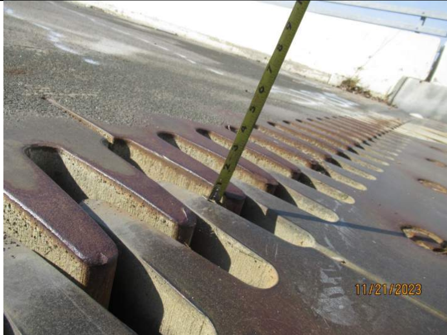
Photo S-127 - [South Abutment] -Detail view showing approach (south) fingers up to 0.75" higher than span (north) fingers in shoulder lanes, into SB right lane, Looking West
