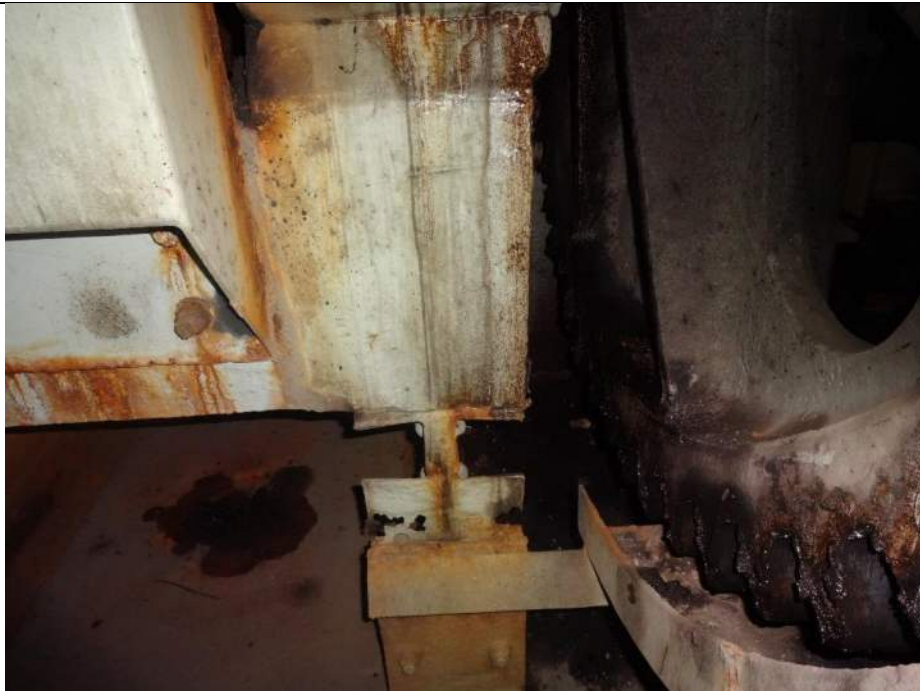
Photo 24 - [NW Corner of North Machinery Room] – There is severe corrosion of fasteners and section loss of base for B2 & B3.
