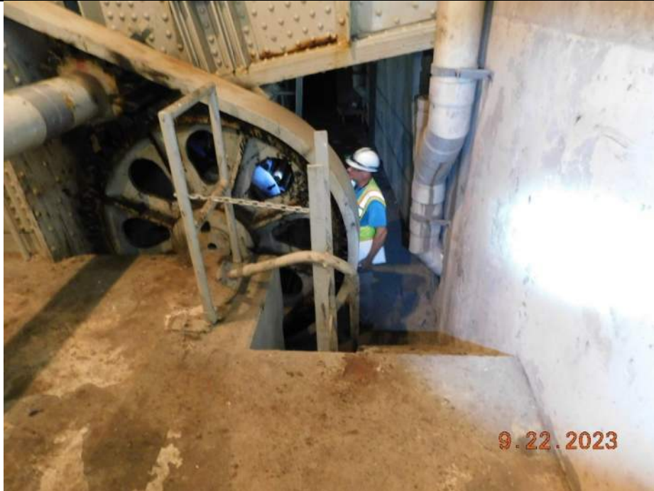
Photo S-365 - [Pier 4 Interior] -Machinery level railing is broken at the east side of G3W, Looking North
