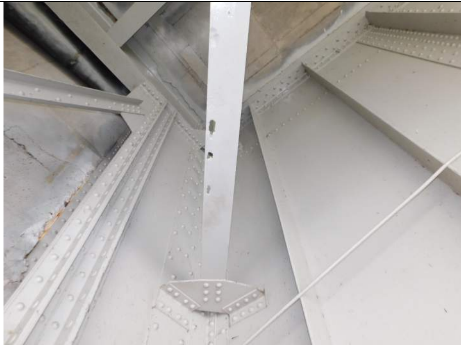
Photo S-208 - [Span 4] -Lower-Level diagonal bracing connection to G2W below FB36S exhibits painted over section loss and several small holes in the flange, Looking Northeast
