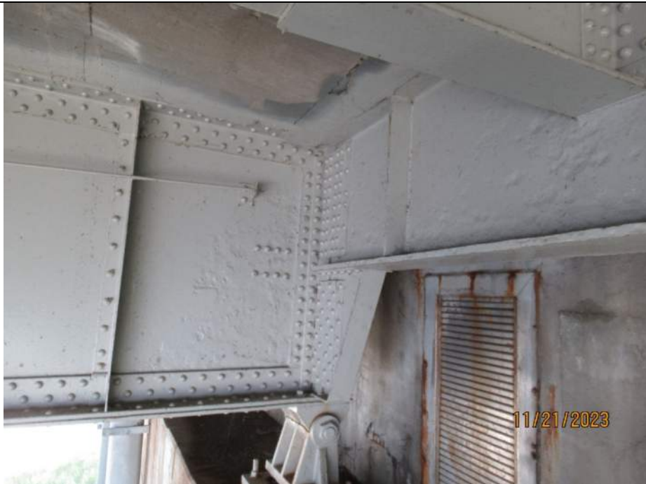
Photo S-174 - [Span 1] -Girder 4W West face at FB0S, scattered section loss up to 0.125" deep across web and bottom flange, floorbeam connection, similar at floorbeam, Looking Southeast
