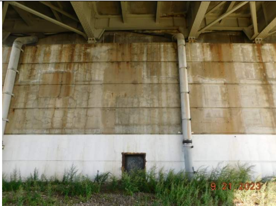
Photo S-274 - [South Abutment] -Abutment stem and back wall view between Girders 3W-5W, Looking South
