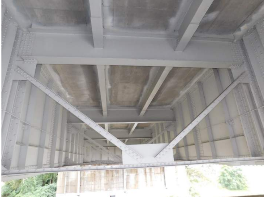
Photo S-173 - [Span 1] -Interior framing between Girders 2W-3W at FB6S, paint in typically good condition throughout, Looking South
