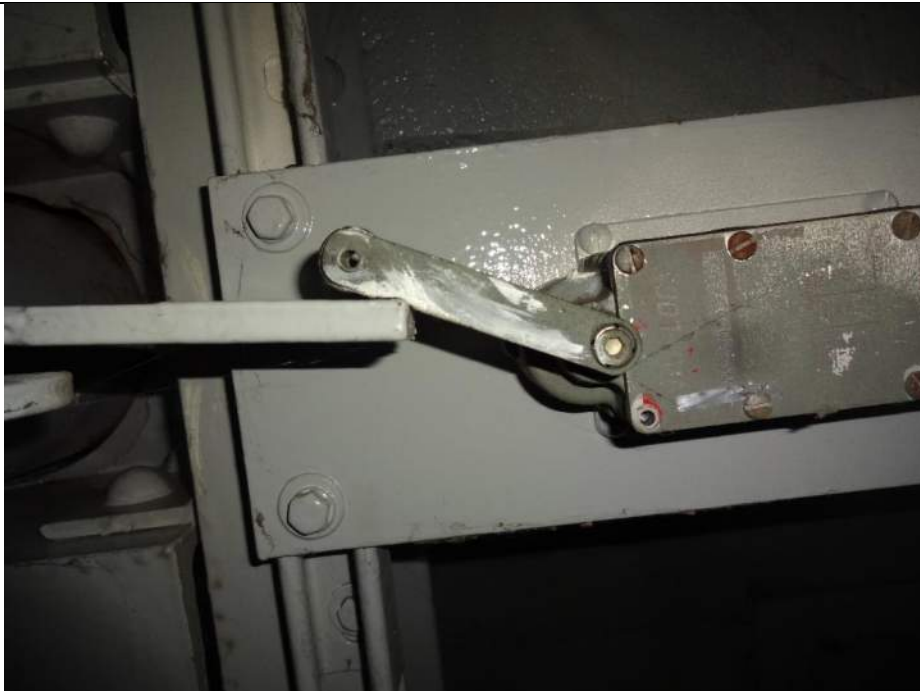
Photo 80 - [NW Swing Gate] – Rollers, though in better condition than SE gate, are misaligned.
