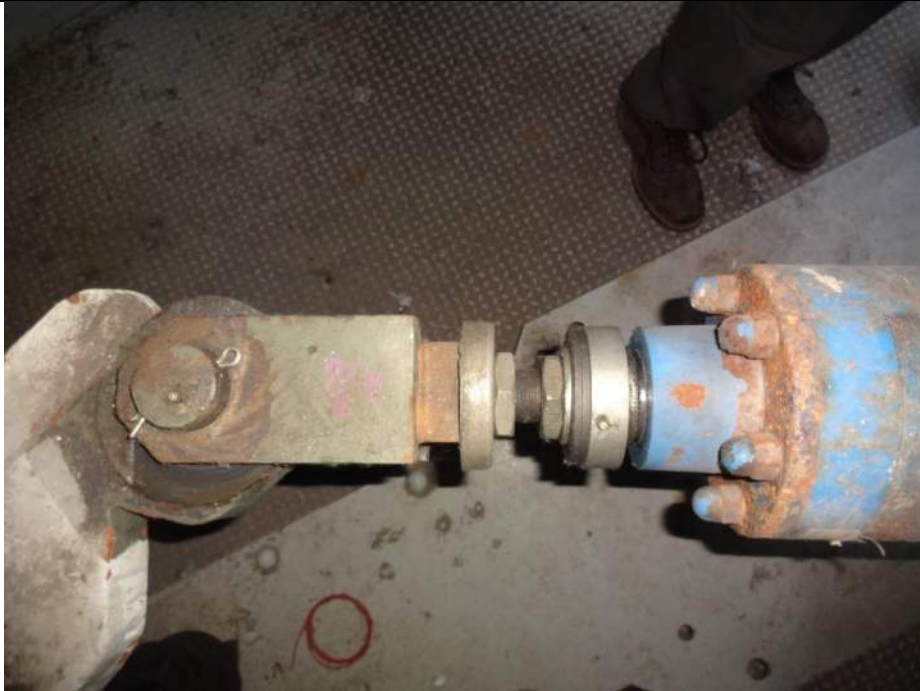
Photo 79 - [NW Swing Gate] - No protective boot is present on swing gate actuator arm.
