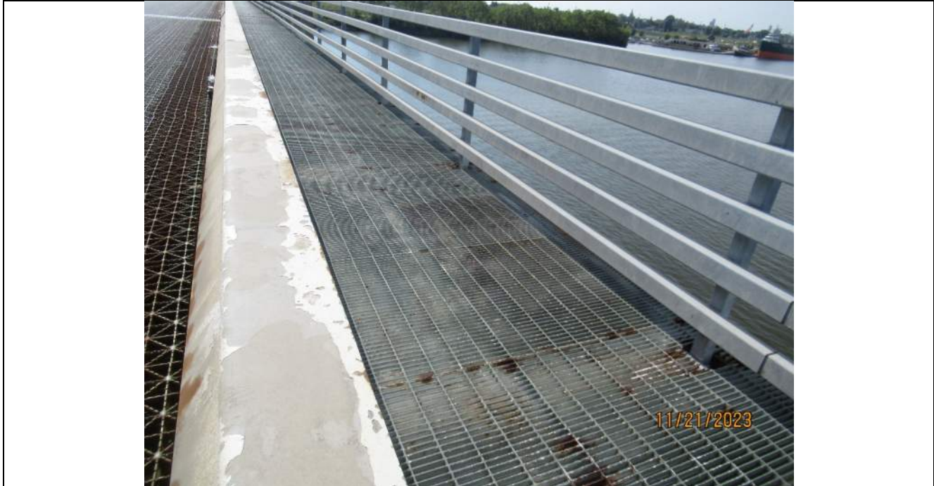
Photo S-109 - [Span 5] -North leaf west sidewalk and railing, typical good condition with spots of corrosion, Looking South
