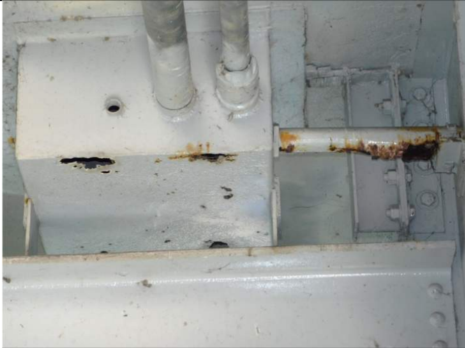
Photo S-331 - [Span 2] -Electrical junction box and conduit above Floorbeam 11S East exterior, holes in box and conduit, Looking North
