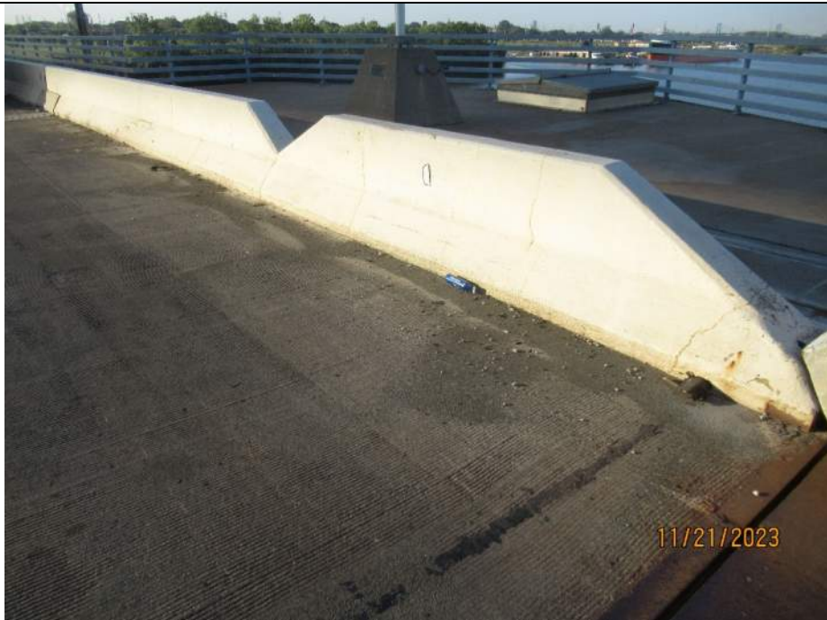
Photo S-90 - [Pier 4 Span] -West roadway barrier, typical vertical cracks, Looking Southwest
