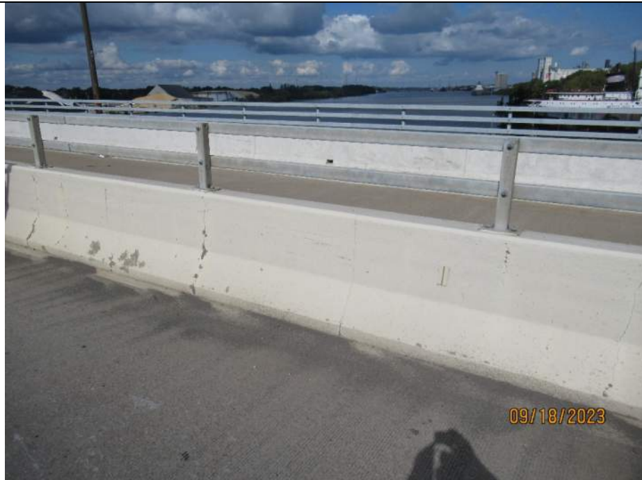
Photo S-82 - [Span 1] -East roadway barrier, typical full height vertical cracking, Looking East
