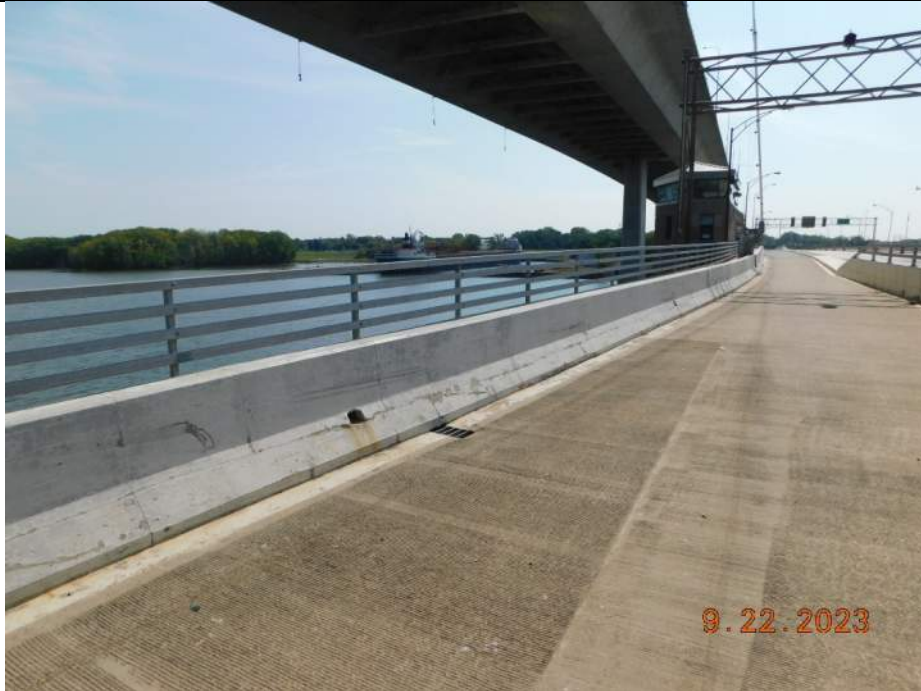
Photo S-95 - [Span 6] -East sidewalk / trail barrier and railing, typical full height vertical cracking, Looking South
