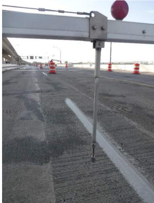
Photo 70 - [NE Traffic Gate] - Gate bumper does not contact the roadway when gate is down.
