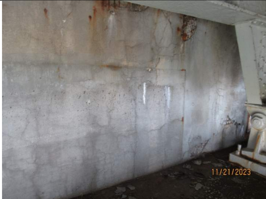
Photo S-275 - [South Abutment] -Abutment backwall at Girder 3W, cracking throughout and minor delamination and shallow spalls, Looking South
