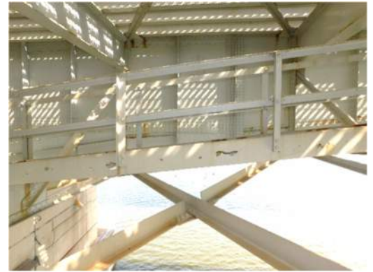
Span 5 North leaf, catwalk channel web holes
