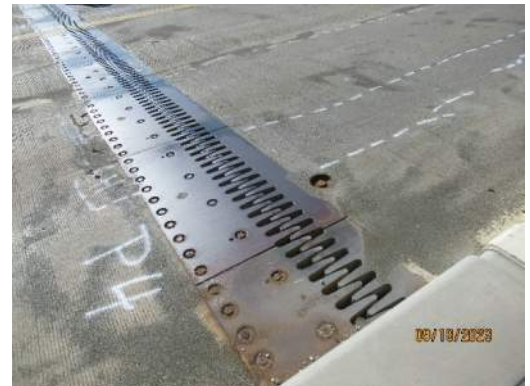
Pier 4 finger joint in NB lanes
