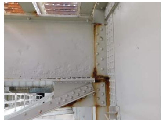
Span 5 K-brace connection plate hole
