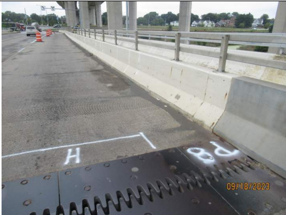
Photo S-98 - [Span 9] -East roadway barrier and top railing, trail / sidewalk barrier and railing in background, typical full height vertical cracking, Looking Northeast
