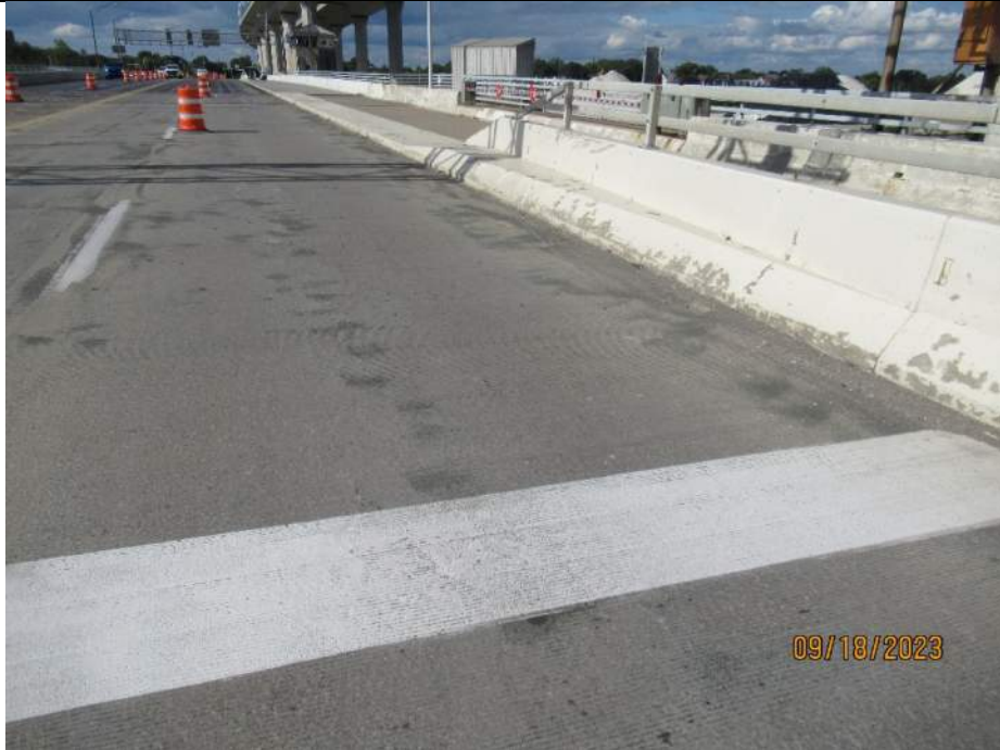
Photo S-47 - [Span 4] -Roadway deck and wearing surface, NB lanes north of mid-span, Looking North
