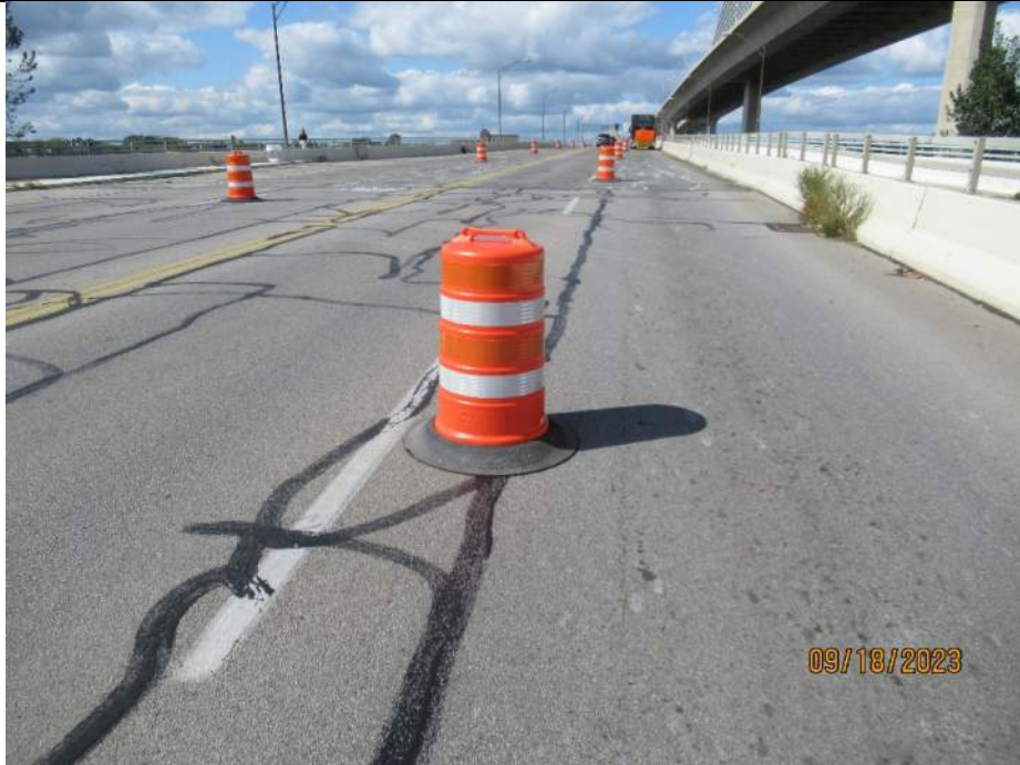
Photo S-9 - [South Approach] -Roadway approach pavement, NB right and left lanes general view, Looking North
