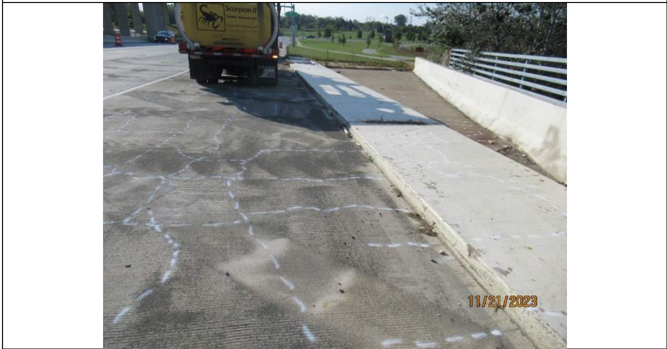
Photo S-18 - [South Approach] -Southwest bridge barrier and raised curb at SB roadway shoulder, Looking South
