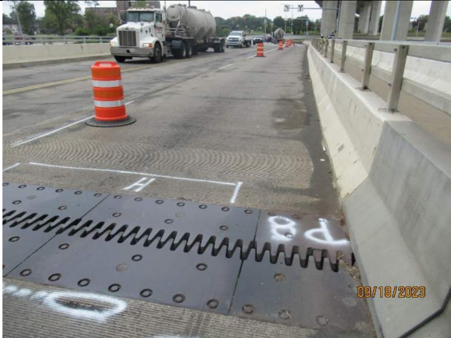
Photo S-65 - [Span 9] -Roadway deck and wearing surface, NB right lane from Pier 8, Looking North
