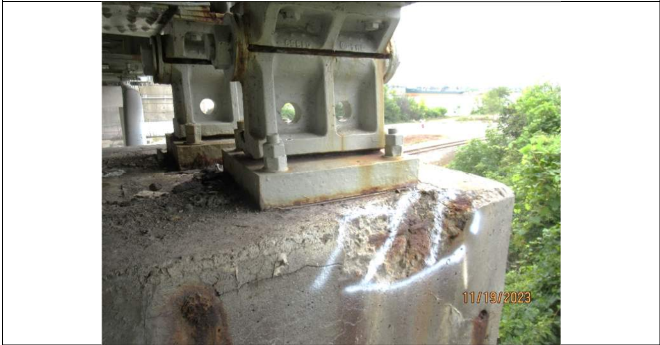
Photo S-312 - [Pier 8] -Pier North face below Bearing 1W, corner spall with exposed rebar, Looking South
