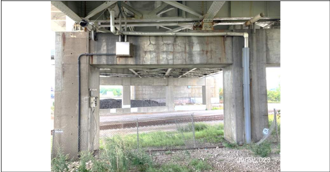
Photo S-152 - [Pier 8] -Drainage troughs are not connected to downspouts at pier and downspouts have missing segments, Looking South
