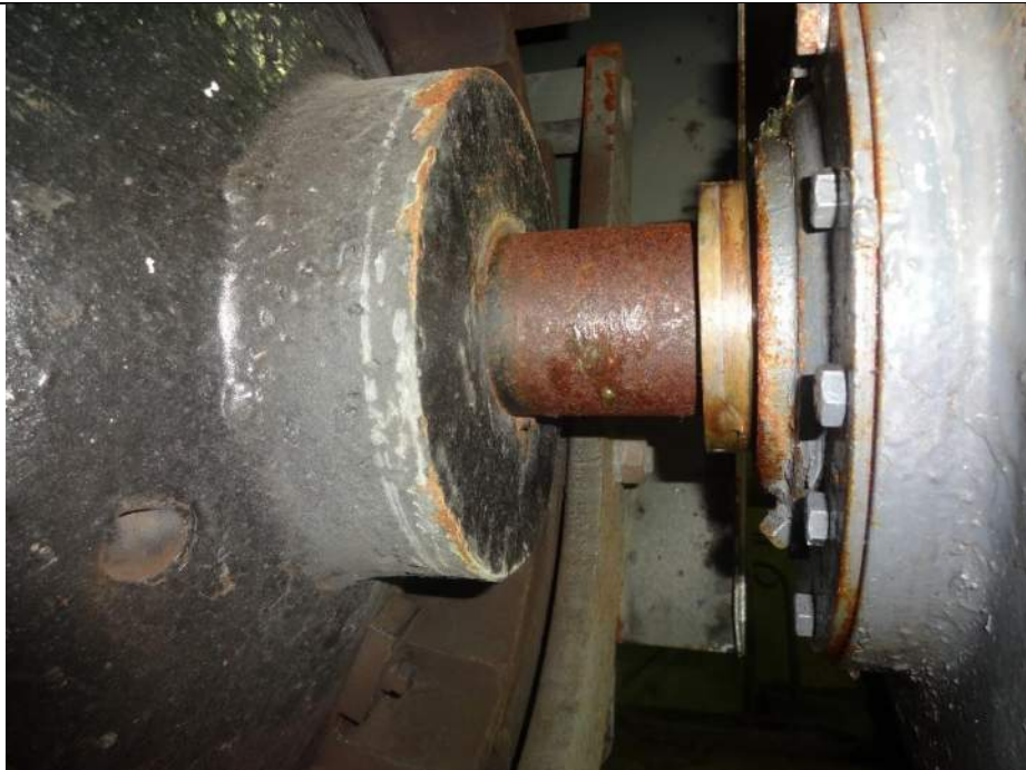
Photo 2 - [North Machinery Room] – Note surface corrosion on motor shafts and hubs.
