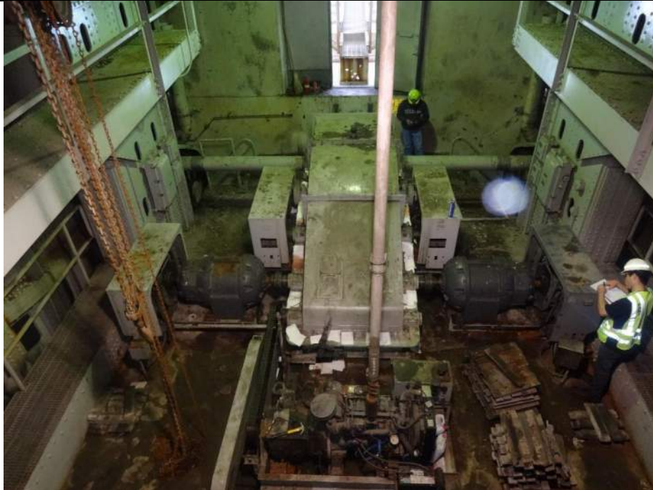
Photo 1 - [North Machinery Room] - Machinery Room Layout
