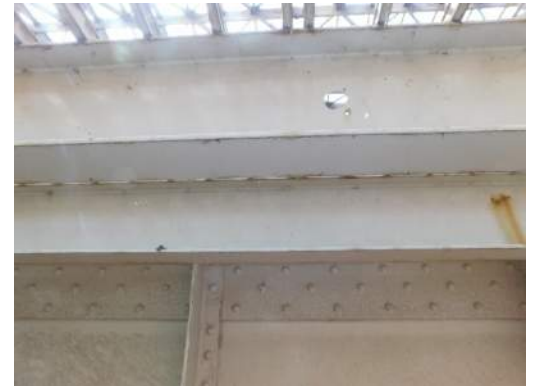
Span 5 North leaf, Stringers 10W + 11W web holes
