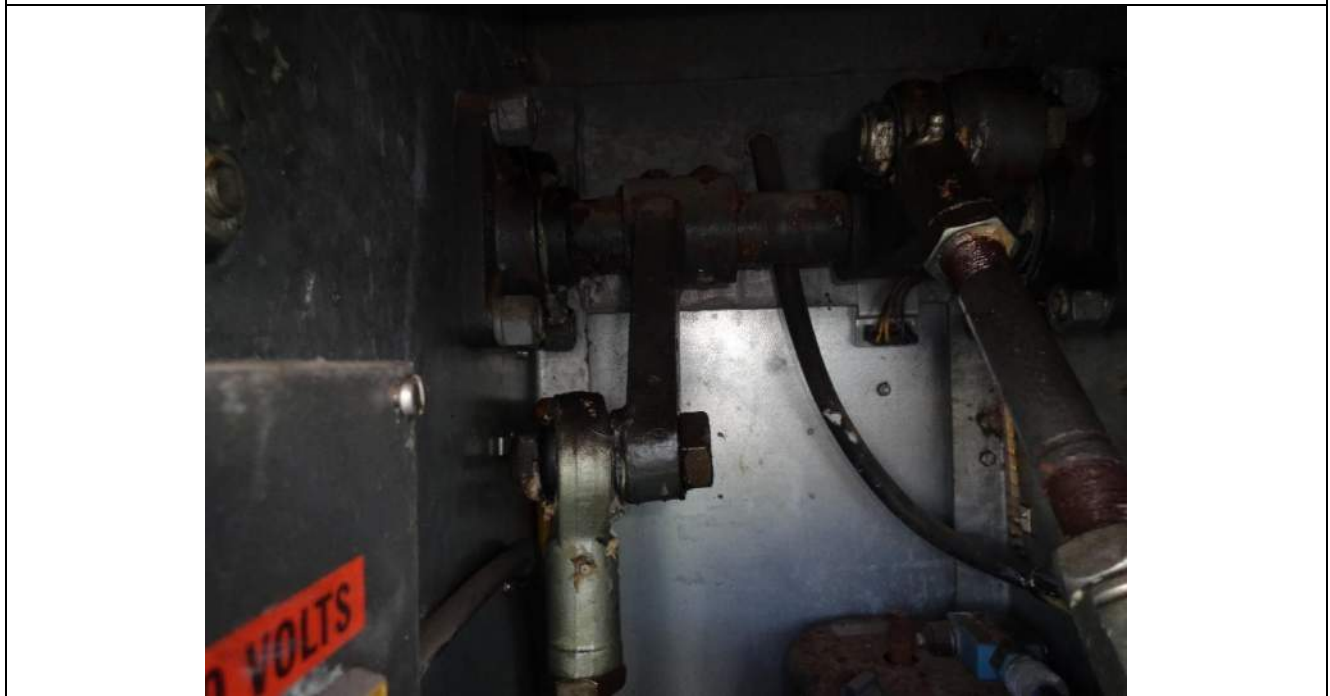
Photo 72 - [SW Traffic Gate] - Levers exhibit slight deformation and misalignment.
