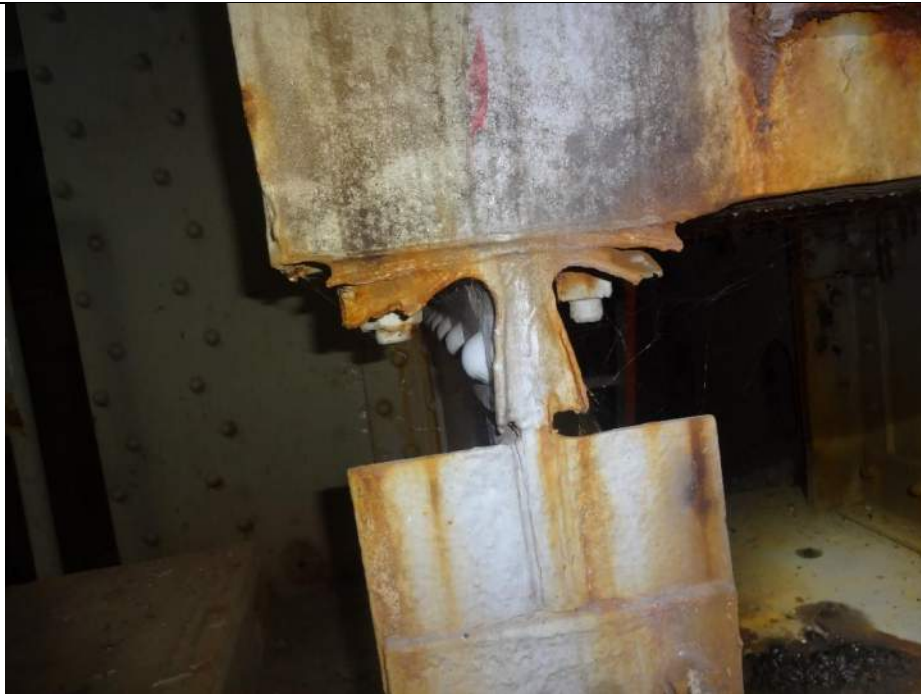
Photo 22 - [NW B1 Bearing] - Pack rust is below base of B1 bearing.
