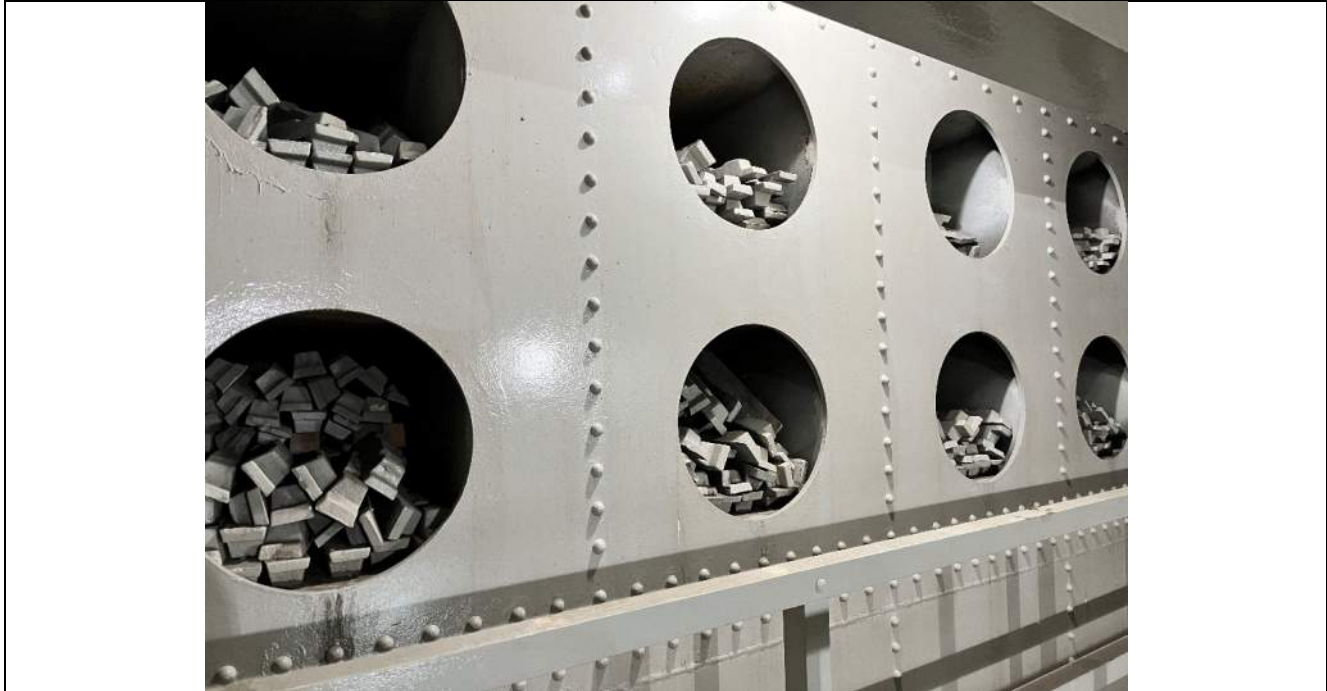
Photo S-363 - [Pier 5 Interior] -Counterweight pockets and blocks detail view, between G3W-G4W, Looking Northeast
