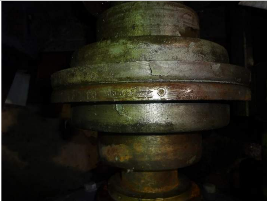
Photo 14 - [North Machinery Room] – Note surface corrosion and paint failure on couplings along with stripped grease plugs.
