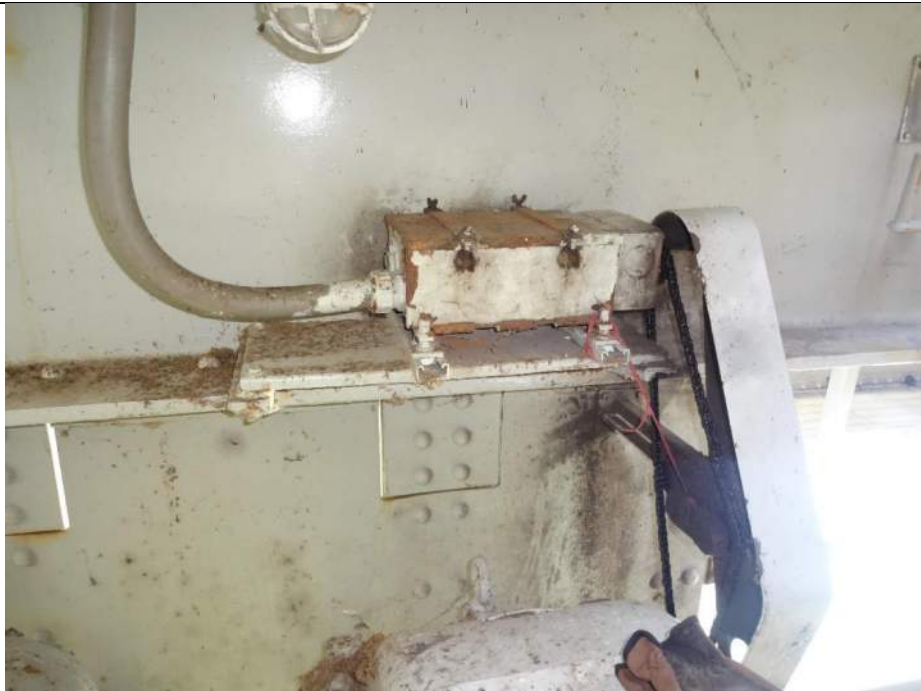
Photo 44 - [RLCS Instrumentation] – Note top wingnuts seized, old oil on chain, tensioner held by wire and heavy corrosion on top surface
