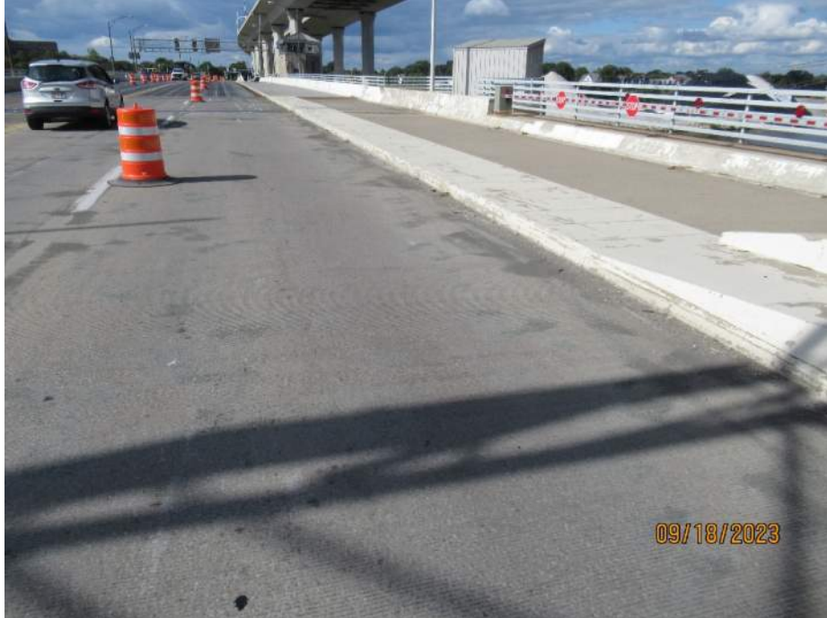
Photo S-105 - [Span 4] -Concrete curb / median island between northbound lanes and mixed use trail, minor scrapes in coating, generally good condition, Looking Northeast
