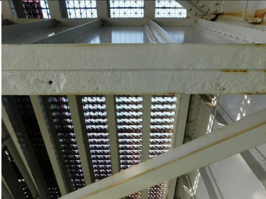
Photo S-221 - [Span 5, South Leaf] -Floorbeam 3s between G1W-G2W, small holes and section loss in bottom flange near G2W, Looking North
