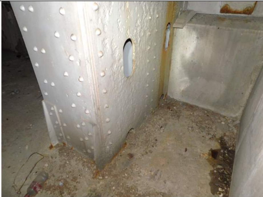
Photo S-352 - [Pier 4 Interior] -Tower 4W West leg at base, exterior of East plate, painted over section loss throughout, Looking Northwest
