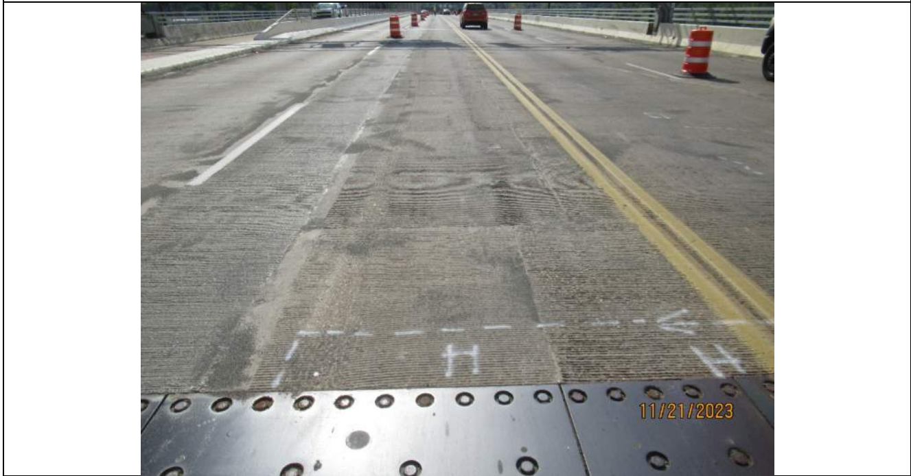
Photo S-50 - [Span 4] -Roadway deck and wearing surface, middle lanes from north end of span, Looking South
