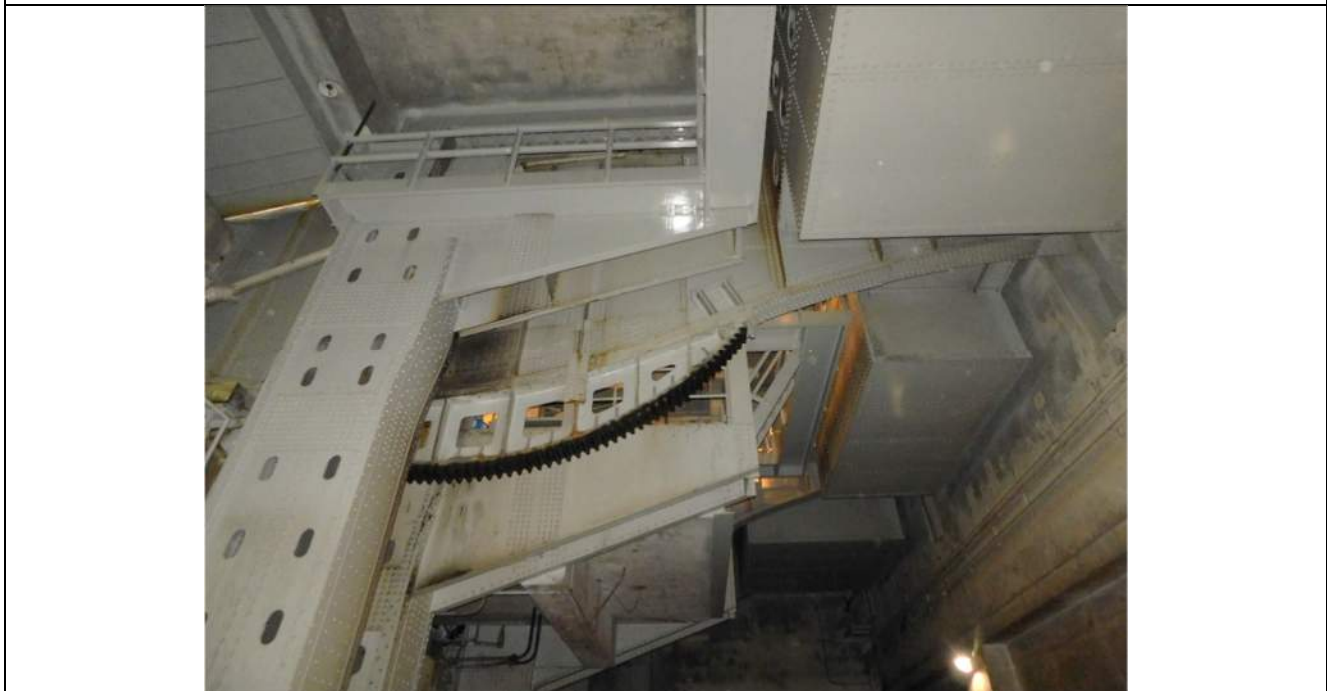
Photo S-360 - [Pier 4 Interior] -Counterweight undersides at girder tails, general view of lower portions at G2W, G3W, Looking East
