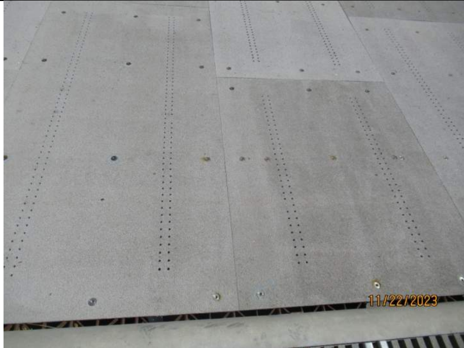
Photo S-61 - [Span 5] -South leaf trail segment, detail view of bolted panel sections in good condition, Looking East
