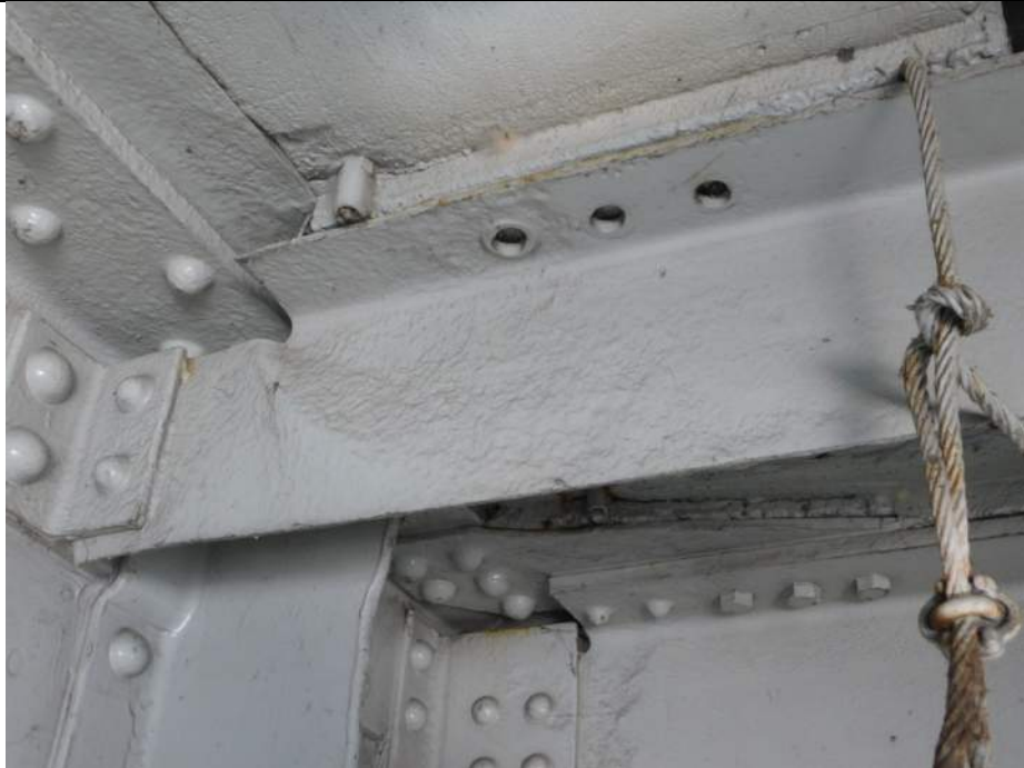
Photo S-205 - [Span 4] -Sidewalk framing member with section loss below deck curb location, minor web buckling and pinhole, between Floorbeams 34S-35S at east sidewalk, Looking Northwest
