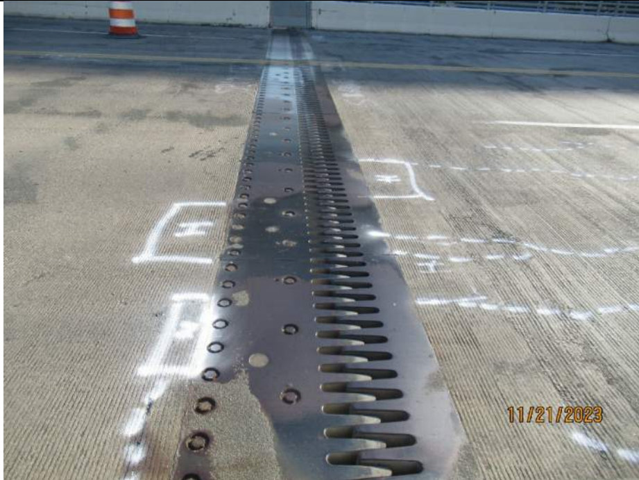
Photo S-125 - [South Abutment] -Abutment reference line finger joint general view in SB lanes, Looking East
