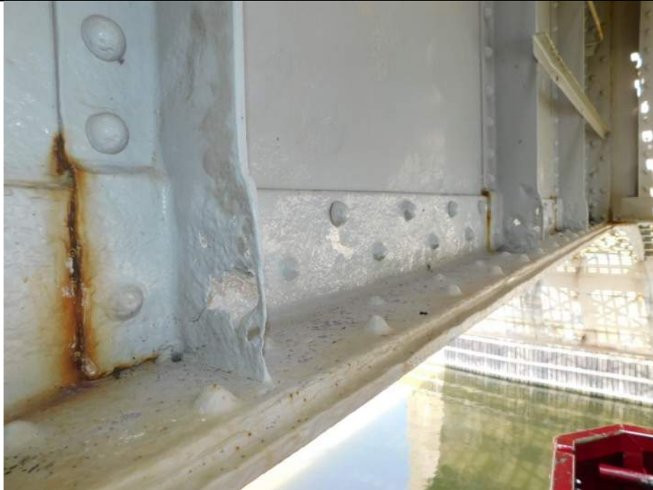
Photo S-211 - [Span 5, South Leaf] -Girder 3W, east BF between FB1s-FB2s, small holes in bases of vertical stiffeners, Looking Northwest
