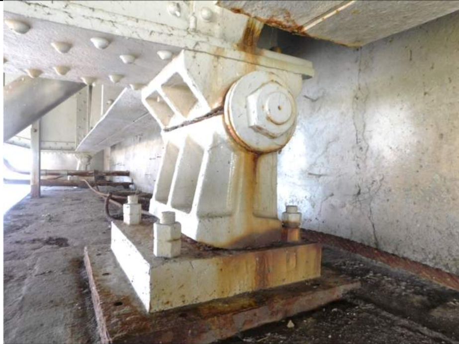
Photo S-261 - [Pier 5] -Bearing 3W at North side of Bascule Pier 5, general view of bearing tilted South in expansion, Looking East
