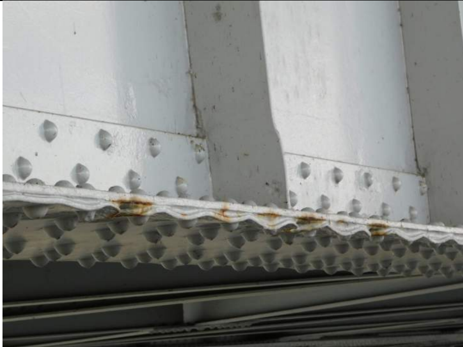
Photo S-179 - [Span 3] -Girder 4W East bottom flange, warping of cover plates due to packing corrosion, detail view FB18-19, Looking Northwest
