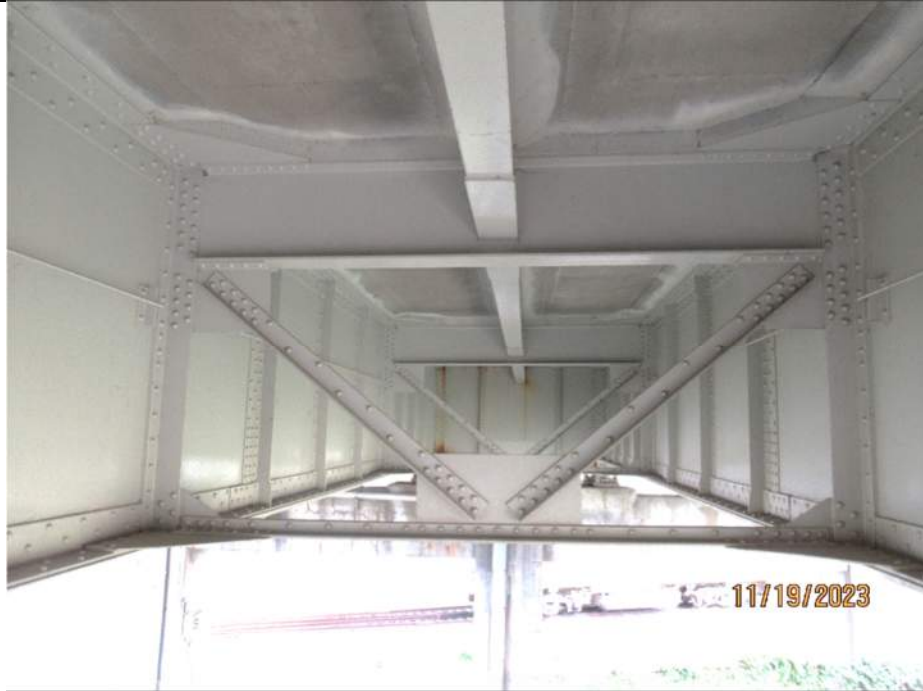
Photo S-271 - [Span 9] -Girders 2W & 3W, Floorbeams 0s-1s-2s, Stringer 3W and secondary framing, general view of paint in good condition, Looking South
