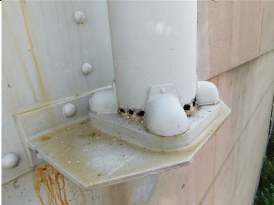
Photo S-315 - [Span 1] -West side light pole at Floorbeam 0S / South Abutment, holes in base of pole across 75% of the perimeter, Looking Southeast
