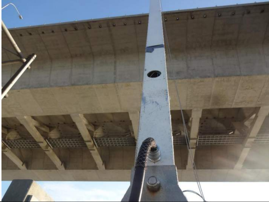
Photo 69 - [NE Traffic Gate] - Cover for electrical access below gate arm is missing.
