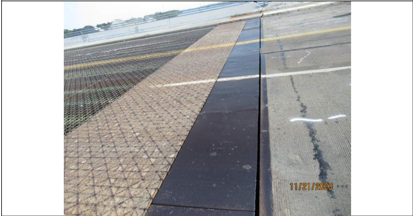
Photo S-142 - [Span 5] -South leaf rear break joint, good condition general view, Looking East
