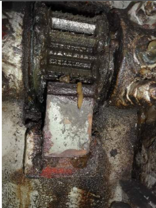
Photo 46 - [NW Inboard Locking Mechanism] – Note paint failure, corrosion, old grease and debris contaminating lubrication in locking mechanism.
