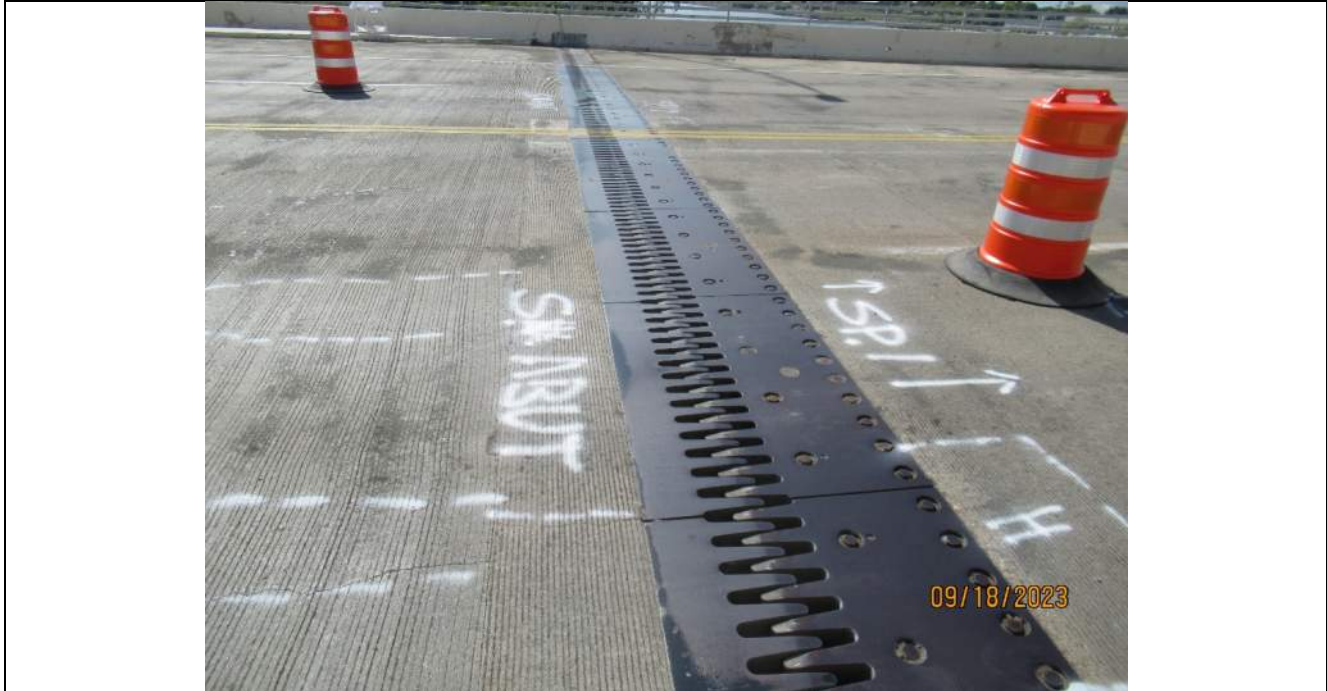
Photo S-121 - [South Abutment] -Abutment reference line finger joint general view from NB lanes, Looking West
