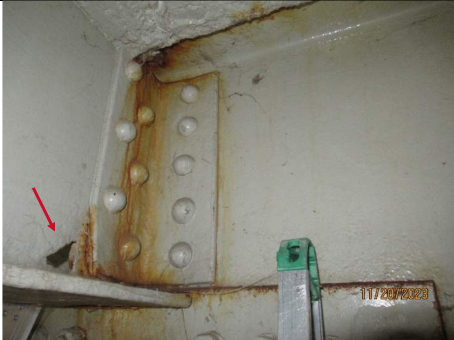
Photo S-203 - [Span 10] -Stringer 3W at the North Abutment exhibits a 2" diameter hole in the lower web at the connection to Floorbeam 11S, Looking North
