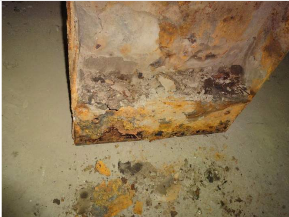
Photo 30 - [North Machinery Room] – Note severely corroded gear cover and failing gear cover gasket.
