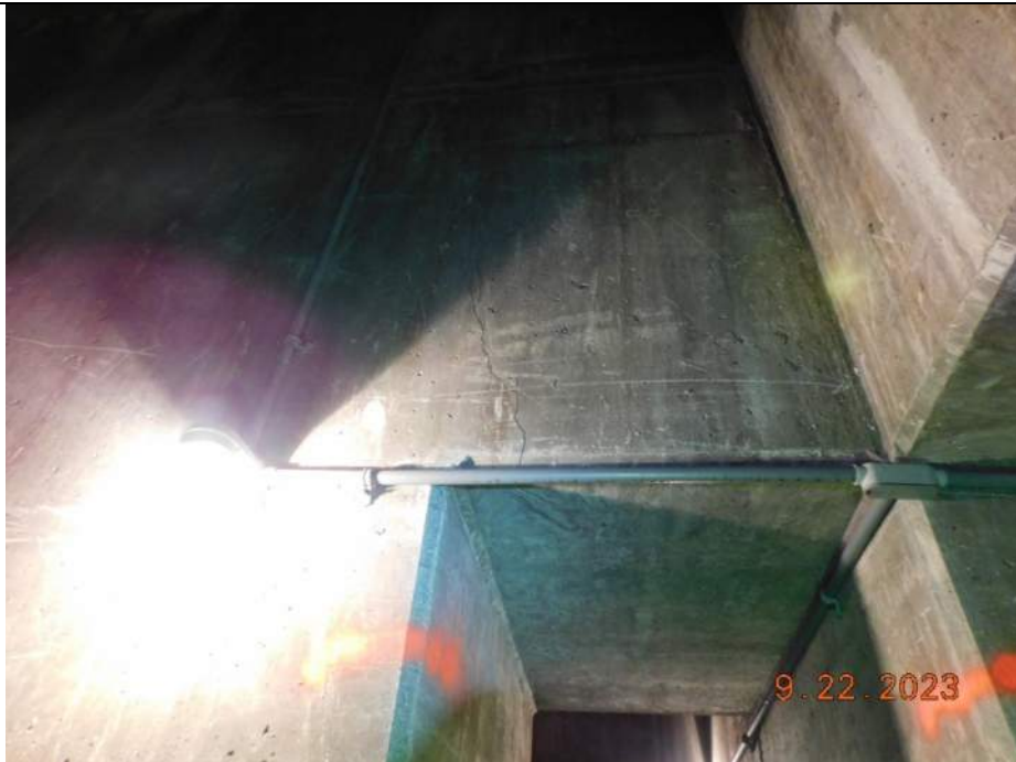
Photo S-342 - [Pier 5 Interior] -Basement Level (Level F), Room 1W, diagonal cracking in interior wall above doorway between north and south sides of west exterior room, Looking North
