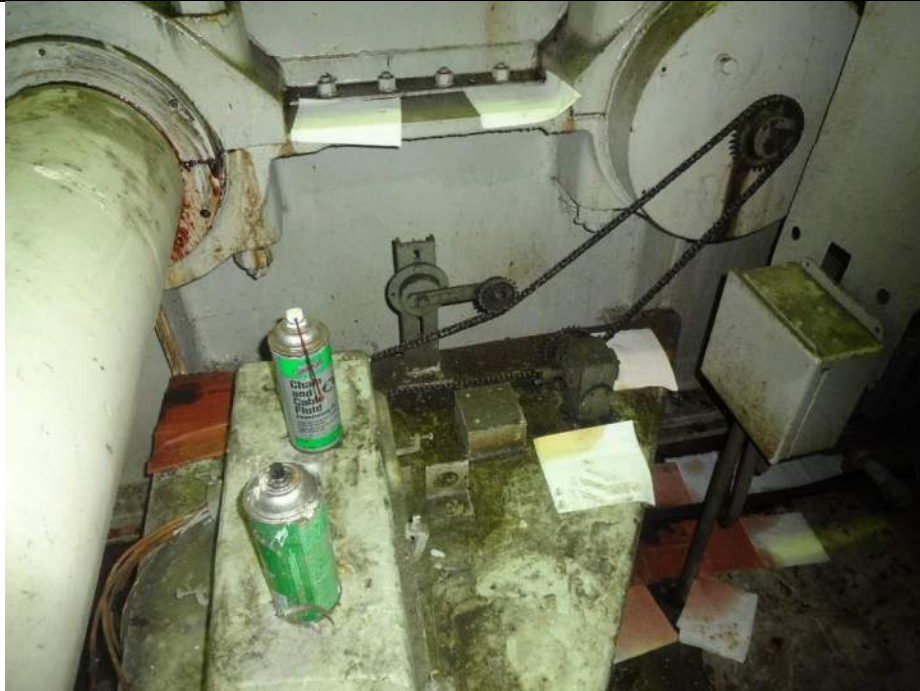
Photo 31 - [North Machinery Room] - Abandoned span drive machinery on North side of bridge is still being maintained.
