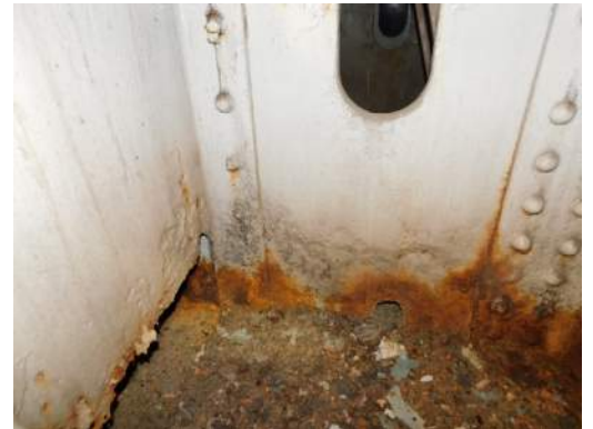
Pier 4 Trunnion Tower 3W, West leg interior at base, typical corrosion and section loss
