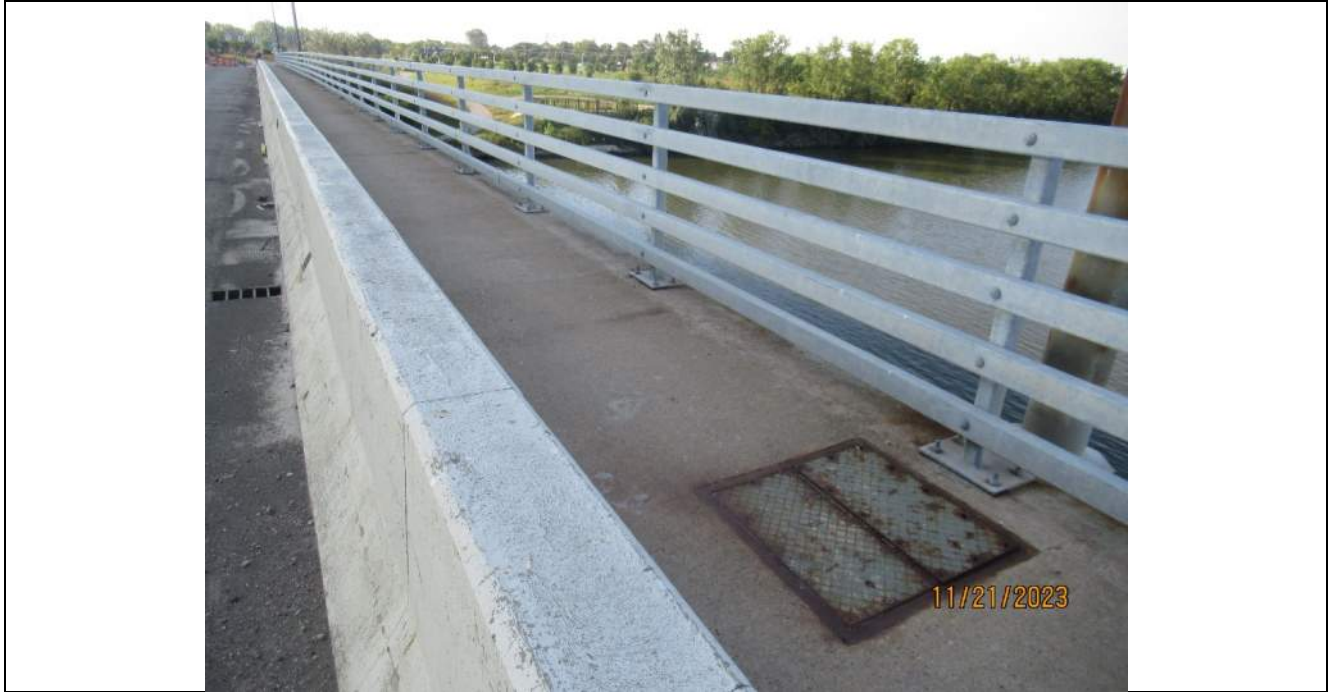
Photo S-104 - [Span 3] -West pedestrian railing and sidewalk, typical good condition, Looking Southwest
