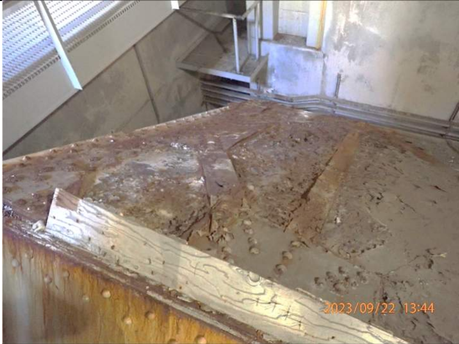
Photo S-361 - [Pier 4 Interior] -Counterweight top at east side (G4W) with moderate corrosion and minor spalling deterioration across the top of the block, Looking Southeast
