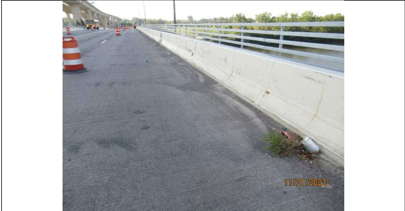
Photo S-87 - [Span 3] -West roadway barrier, typical minor impact scrapes and vertical cracking, Looking Southwest
