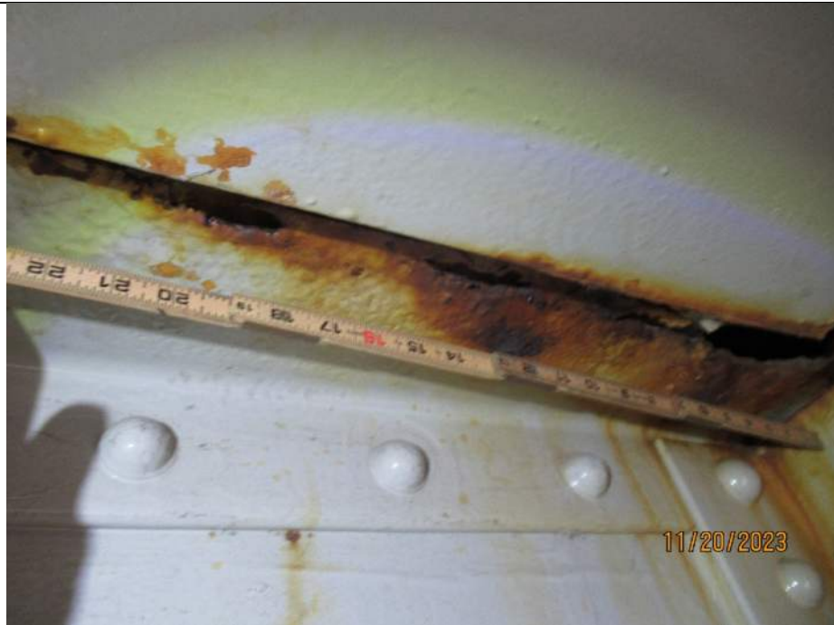
Photo S-193 - [Span 8] -Floorbeam 20S, south top flange angle horizontal leg with heavy section loss for 3 ft lengths on either side of Stringer 3W, Looking North
