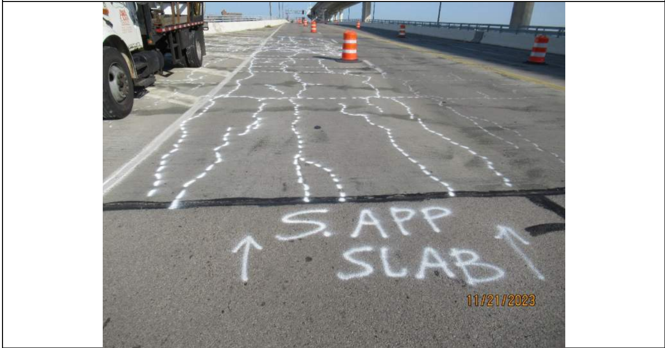
Photo S-16 - [South Approach] -Approach slab HPR joint with approach pavement, SB lanes, Looking North
