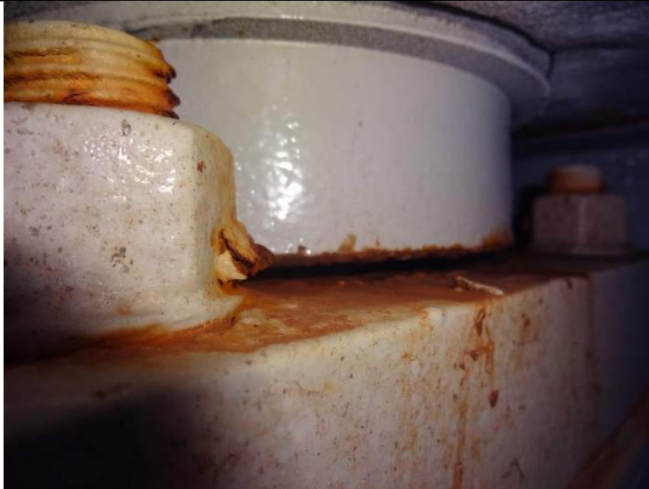
Photo 37 - [NW Outboard Live Load Shoe] - Minor surface corrosion is evident on contacting surface of live load shoes as well as an 1/8" gap.
