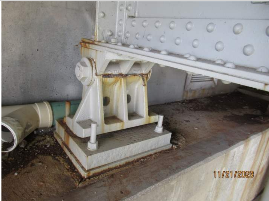
Photo S-254 - [South Abutment] -Bearing 4W, typical minor rust stains and bleeding corrosion, Looking South
