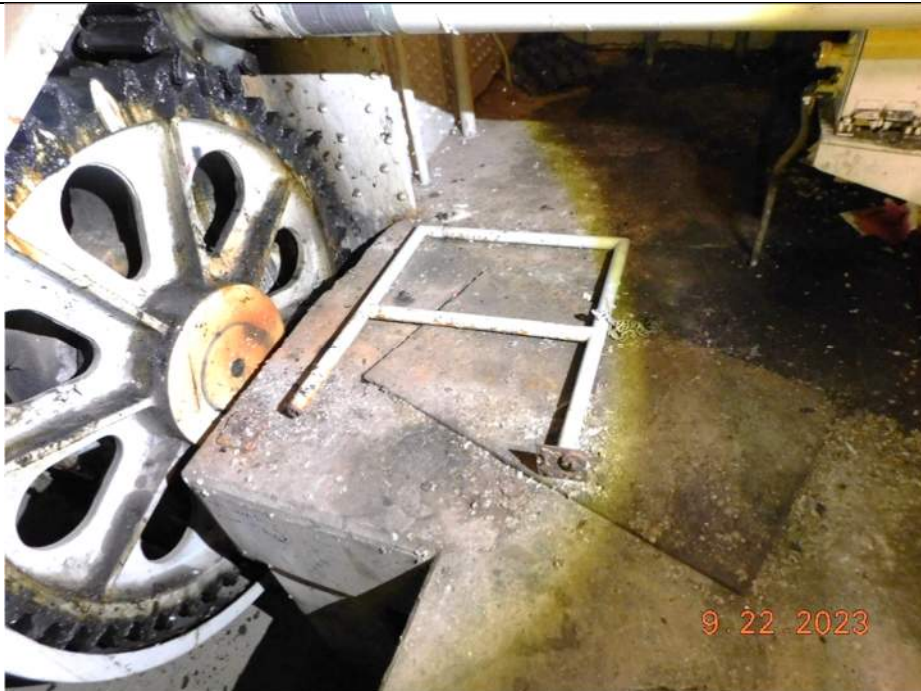
Photo S-366 - [Pier 5 Interior] -Machinery level railing is broken at the west side of G3W, Looking West
