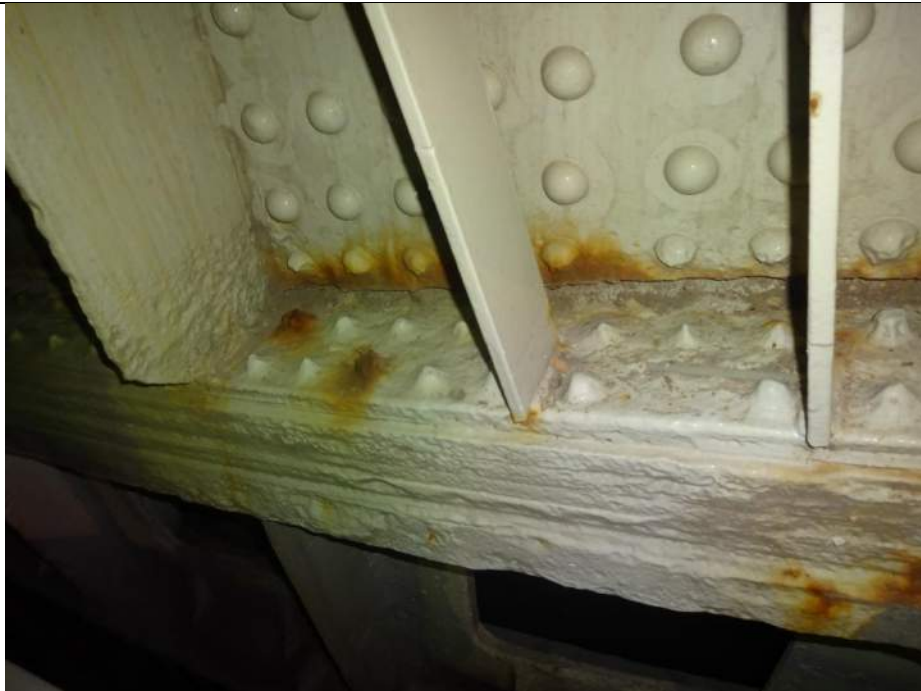
Photo 28 - [NW Rack Segment] - Severe corrosion and section loss appears to be painted over on rack segment fasteners.
