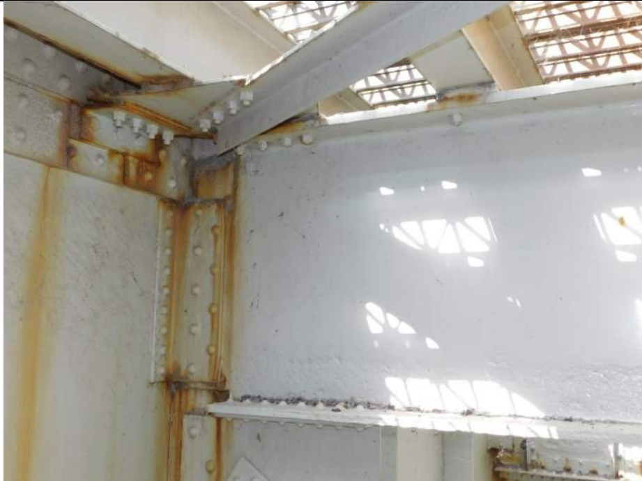
Photo S-231 - [Span 5, North Leaf] -Floorbeam 6n at G2W, typical lower web and bottom flange section loss including rivet head section loss, pack rust at connection and repaired upper diagonal connection, Looking North
