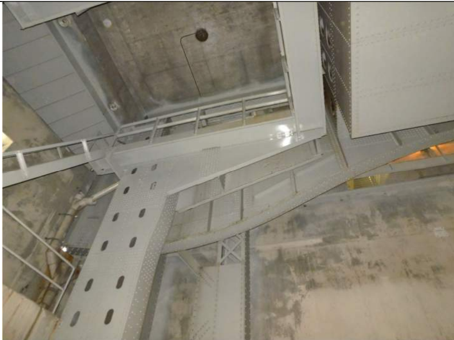
Photo S-350 - [Pier 4 Interior] -Trunnion Tower 4W general view of upper portion of paired tower legs and bascule girder, Looking Northeast
