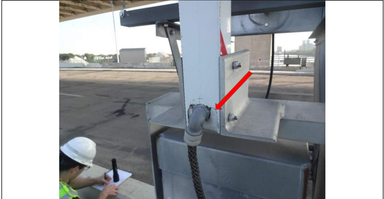
Photo 71 - [SW Traffic Gate] - Gate arm has crack at base where conduit inlet is located.
