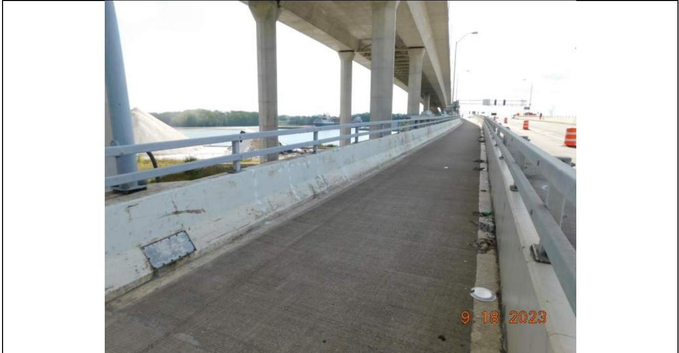
Photo S-101 - [Span 10] -East sidewalk / trail barrier and top railing, typical full height vertical cracking, Looking Southeast
