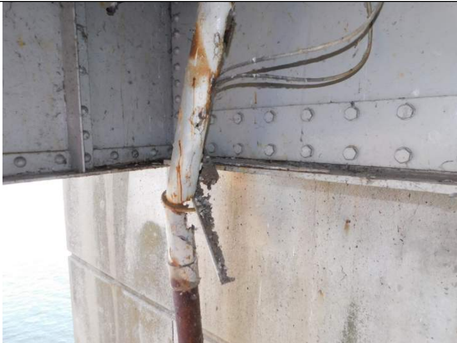
Photo S-334 - [Span 6] -Electrical conduit exhibits 100% SL and a broken support angle at connection to East exterior FB0S with exposed wiring, Looking Southeast
