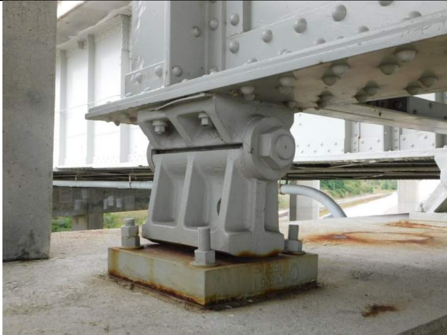
Photo S-263 - [Pier 6] -Bearing 5W, West exterior girder bearing at pier, moderate blister and bleeding corrosion around masonry plate and at lower rocker, Looking North
