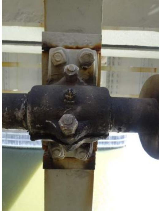
Photo 55 - [NW Span Lock Bearings] – Note top two bolts on bearing using mismatched hardware: one hex nut and one square nut.
