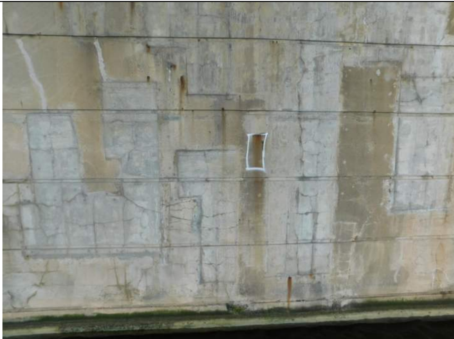
Photo S-296 - [Pier 4] -Pier South face, detail view of widespread patch and crack repairs, cracking in and around repair areas, Looking Northeast
