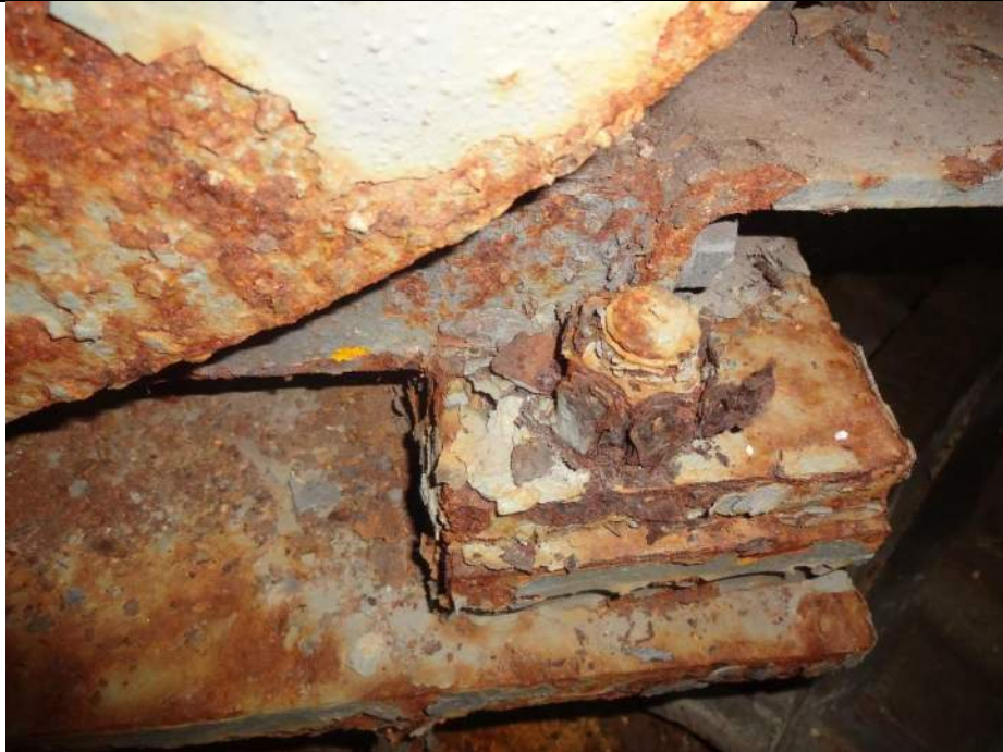
Photo 9 - [North Machinery Room] – Note minor paint failure, surface corrosion, corrosion on the base, corrosion on fasteners and seized bolts on both the motor brakes on the North side.
