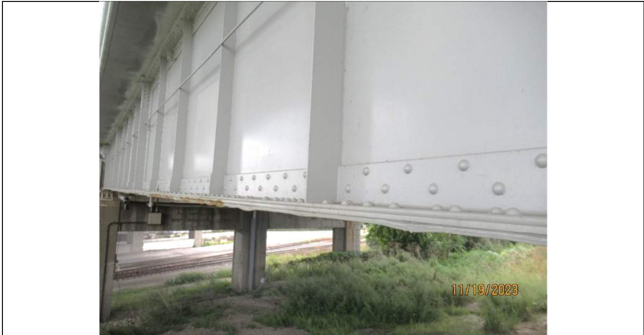
Photo S-185 - [Span 9] -Girder 4W east bottom flange cover plate warping due to up to 1" thick pack rust between plates, Looking Southwest
