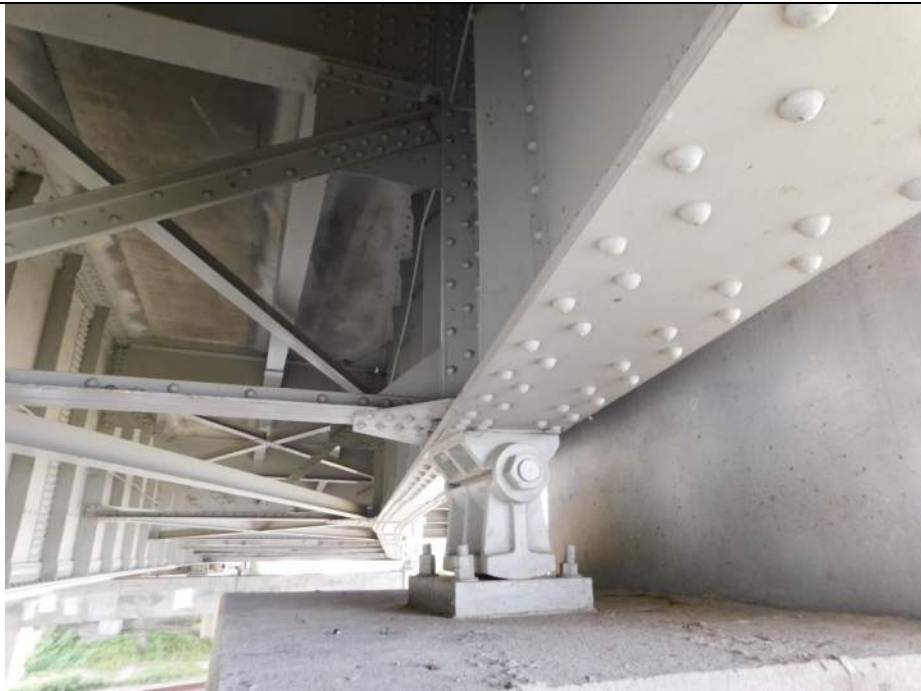
Photo S-264 - [Pier 6] -Bearing 7W, East flare girder bearing at pier, general view in good condition, Looking North
