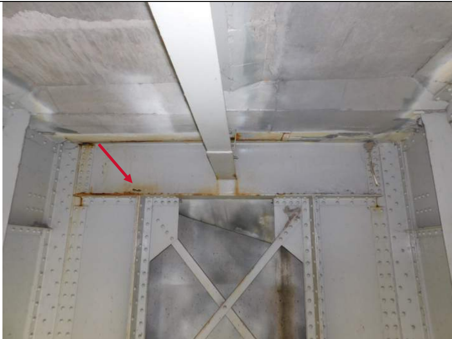
Photo S-190 - [Span 6] -Floorbeam 0S at Pier 5 between Girders 2W and 3W, painted over section loss at lower web with holes, Looking South
