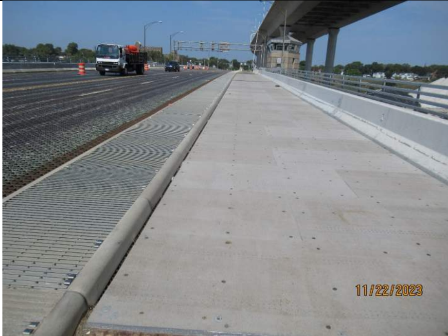
Photo S-59 - [Span 5] -South leaf NB lanes, raised curb and panel-covered trail segment, general view of elements in good condition, Looking North
