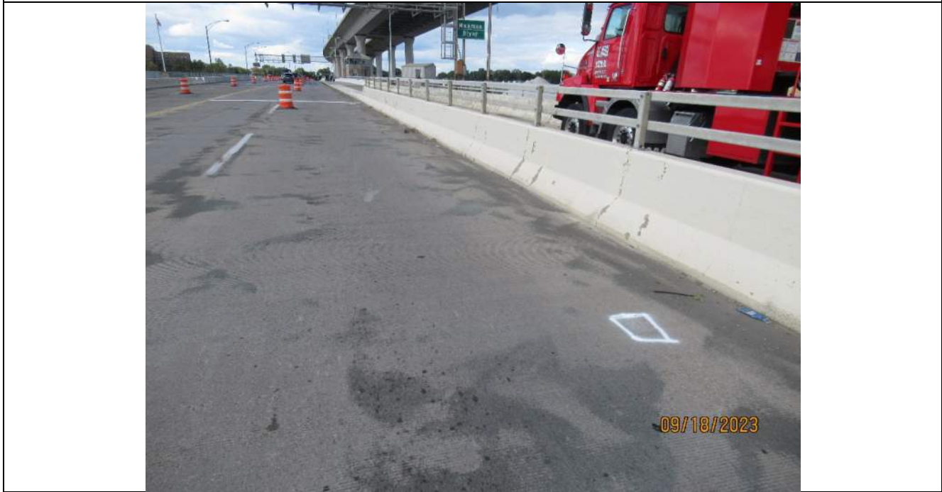
Photo S-88 - [Span 4] -East roadway barrier, typical full height vertical cracking, Looking Northeast
