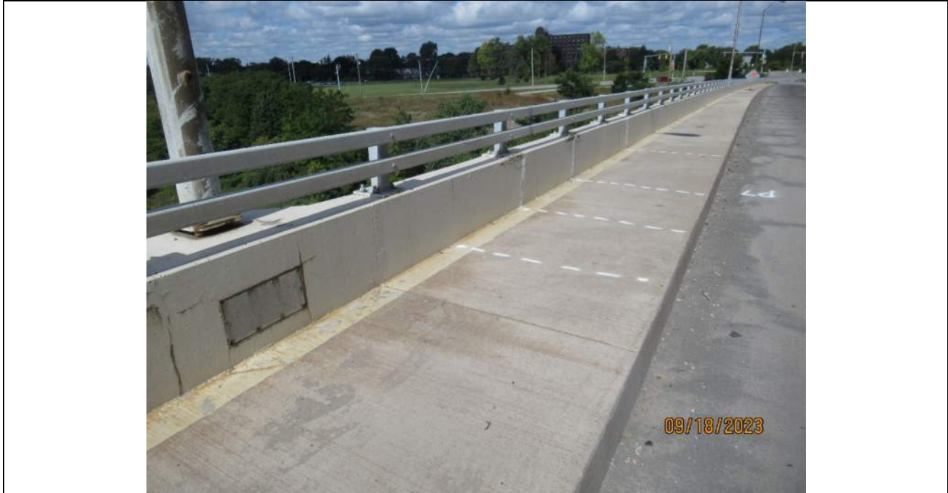
Photo S-117 - [Span 7 & 8] -West sidewalk, barrier and railing, minor transverse and vertical cracking, Looking North
