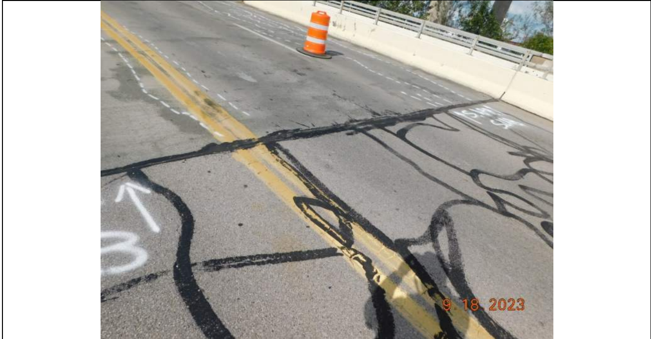
Photo S-17 - [South Approach] -Approach slab HPR joint with approach pavement, NB lanes, Looking Northeast
