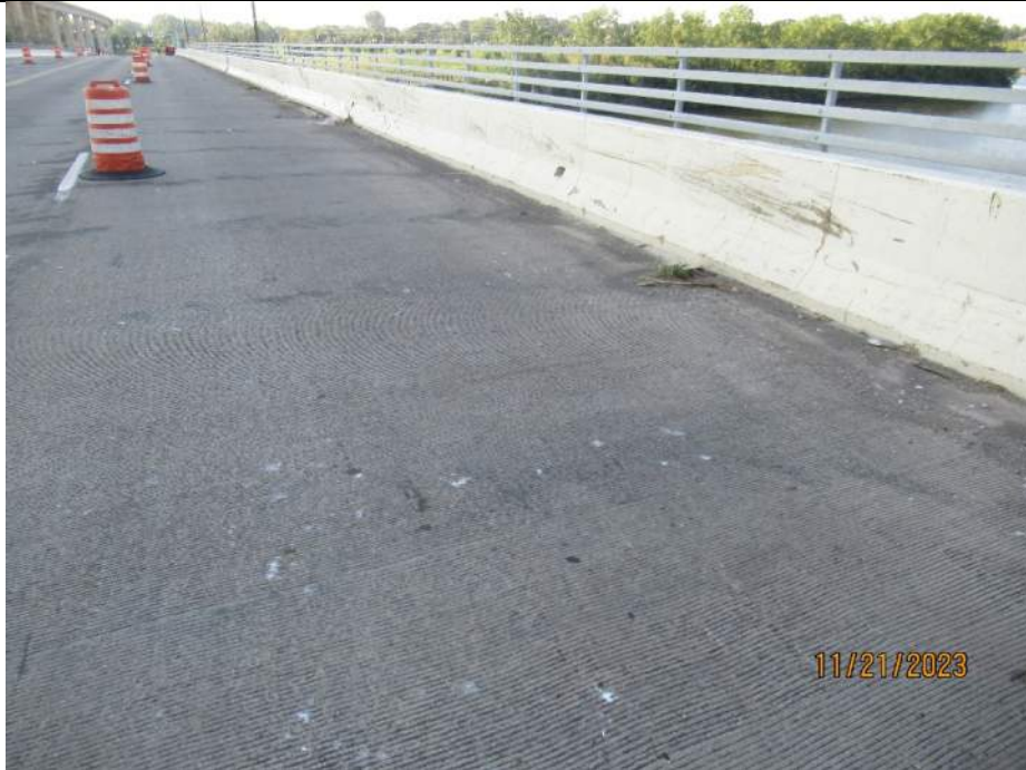
Photo S-89 - [Span 4] -West roadway barrier, typical full height vertical cracking, Looking South
