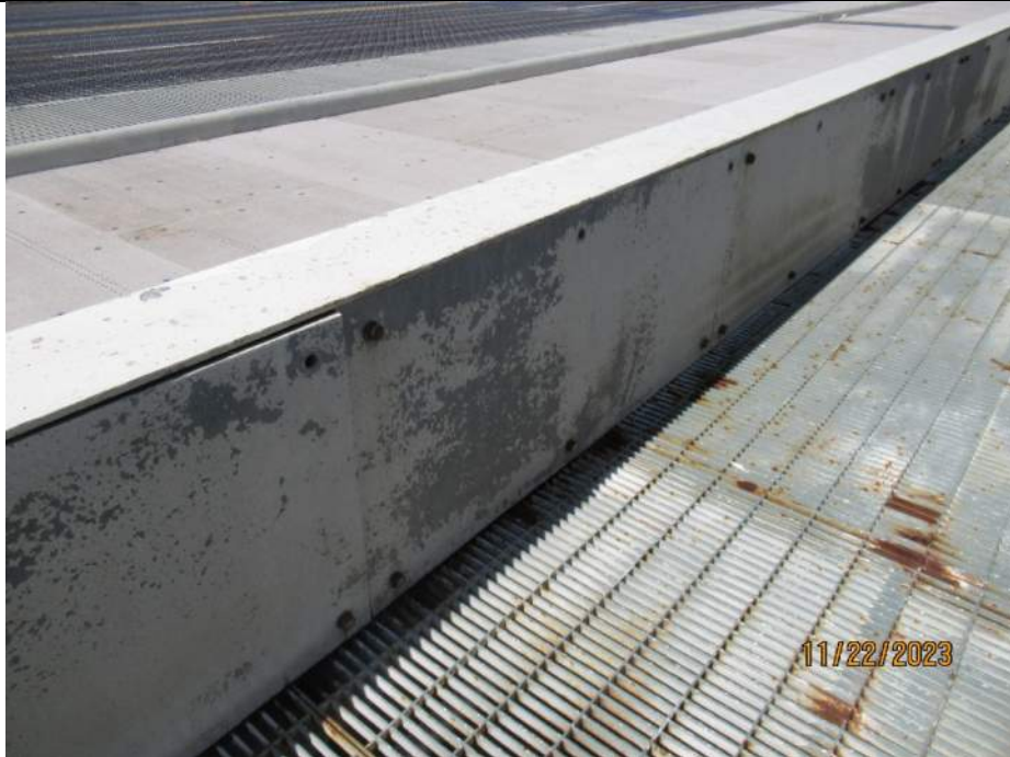
Photo S-93 - [Span 5] -South leaf East roadway / trail steel barrier, East side, scattered missing connection bolts for vertical plate, Looking Northwest
