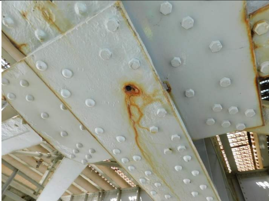
Photo S-215 - [Span 5, North Leaf] -Girder 3W, bottom flange at FB2n, one missing bolt at repaired diagonal bracing connection plate, Looking Northwest
