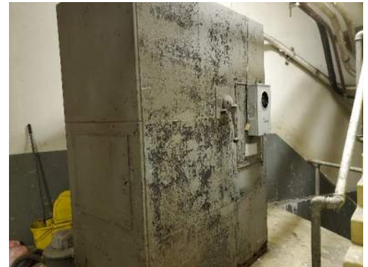
Photo E1: Abandoned Equipment in the South Pier
