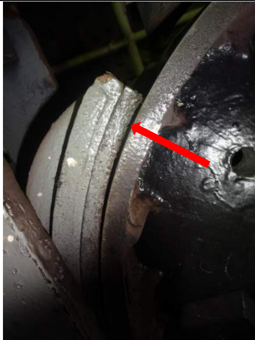
Photo 10 - [NW Motor Brake] – Note poor brake pad contact.
