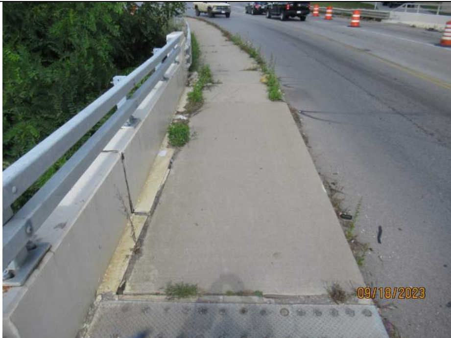
Photo S-26 - [North Approach] -Northwest sidewalk vegetation growth throughout, Looking North
