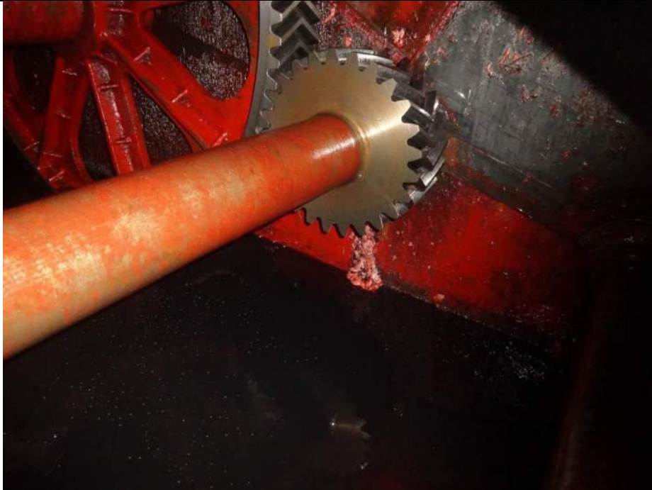
Photo 17 - [North Machinery Room] - Oil is contaminated in central gear boxes.
