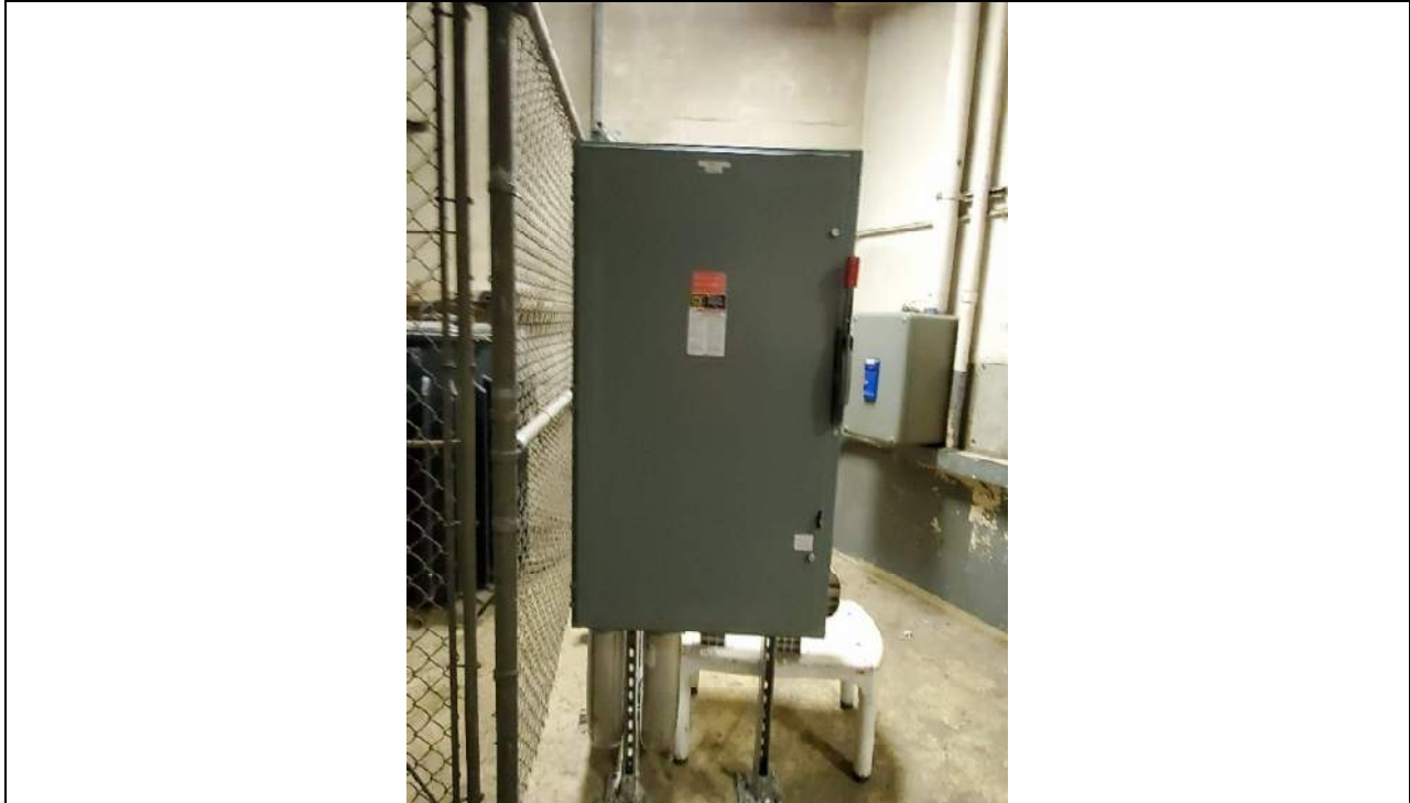
Photo E-03: Service Entrance Disconnect near the Medium Voltage Transformers
