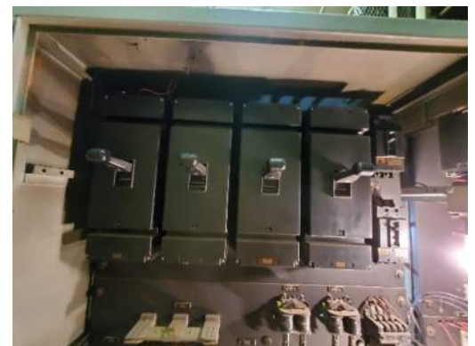
Photo E8: 1950s Circuit Breakers
