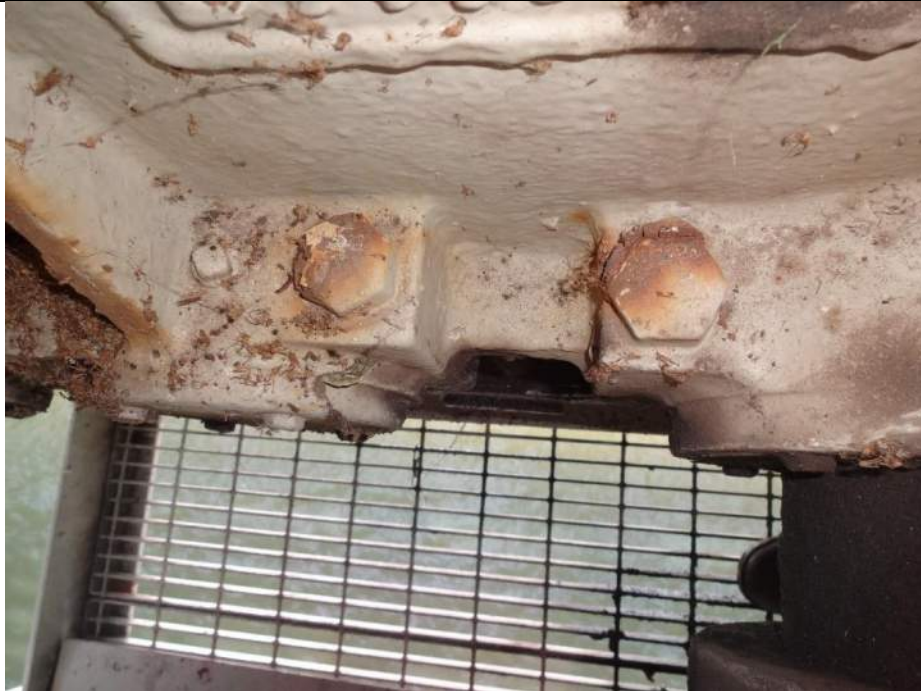
Photo 43 - [Span Lock Reducer] - Isolated corrosion is on fasteners on reducer housing.
