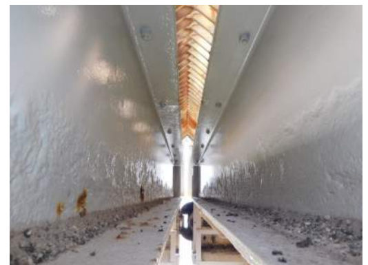
Span 5 FB0s + FB0n, lower web SL below joint, debris accumulation
