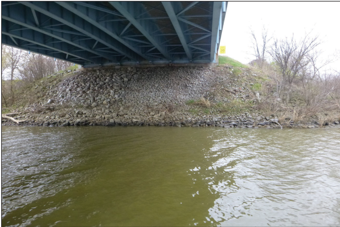
Photograph No. 4: View of the North Embankment at the Structure, Looking North.
