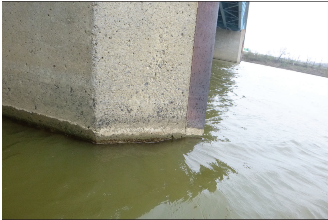
Photograph No. 19: View of the Typical Concrete Condition at the Waterline, Looking South.
