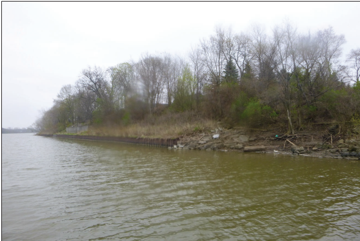
Photograph No. 8: View of the South Embankment Downstream of the Structure, Looking South.
