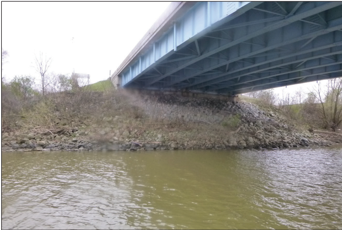
Photograph No. 7: View of the South Embankment at the Structure, Looking Southwest.
