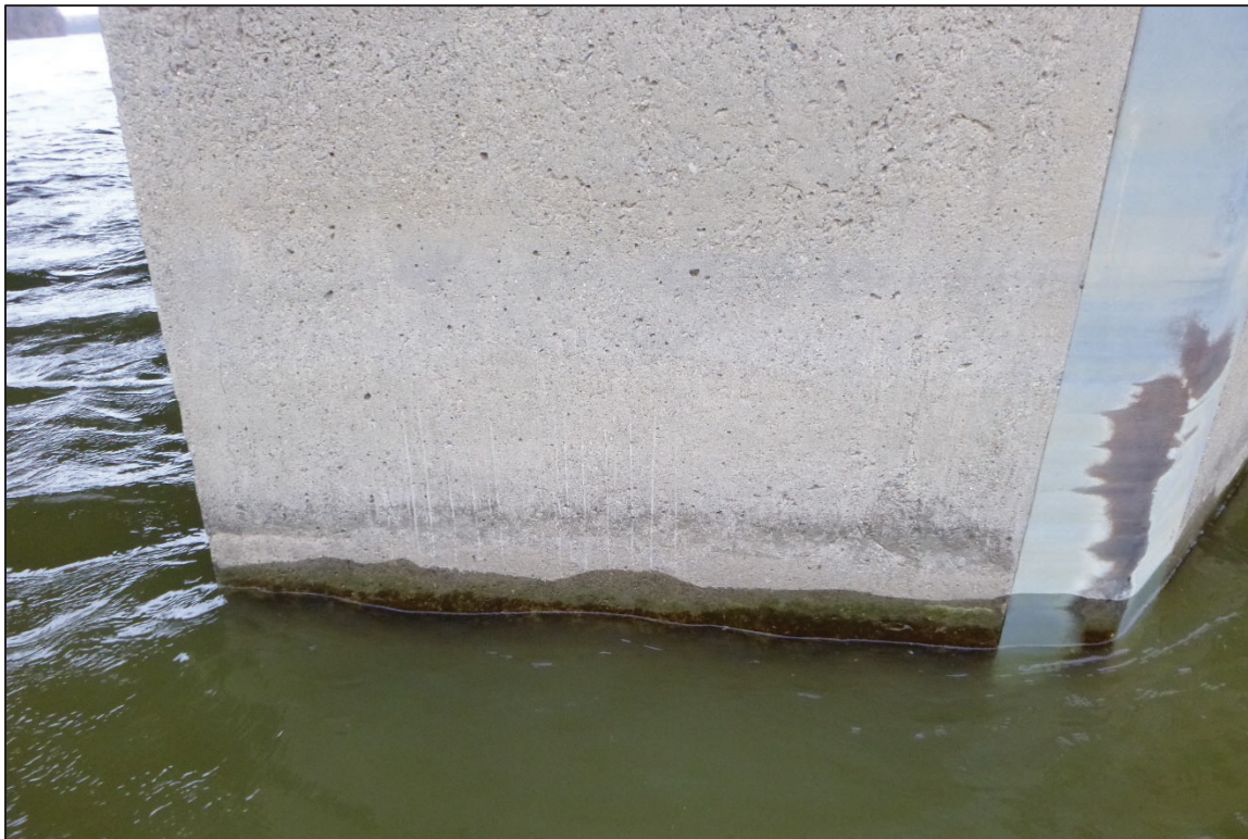
Photograph No. 22: View of the Typical Concrete and Steel Condition at the Waterline on the Upstream Nose of Pier 6, Looking East.
