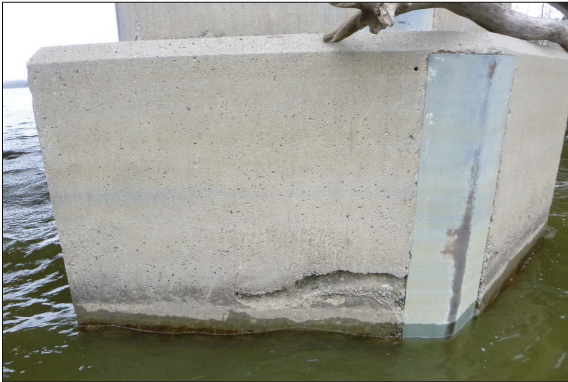
Photograph No. 15: View of the Spall on the Upstream Nose of Pier 3, Looking East.
