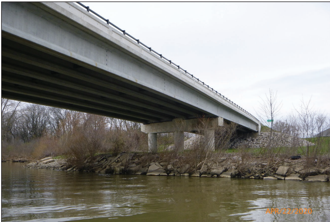
Photograph No. 4: View of the North Embankment at the Structure, Looking Northwest.
