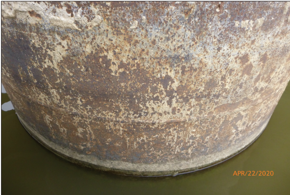
Photograph No. 29: View of the Typical Steel Condition at the Waterline on the Upstream Nose of Bent 1, Looking East.
