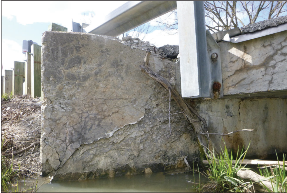
Photograph No. 11: View of Spalling on the South End of Abutment 1, Looking Northwest.
