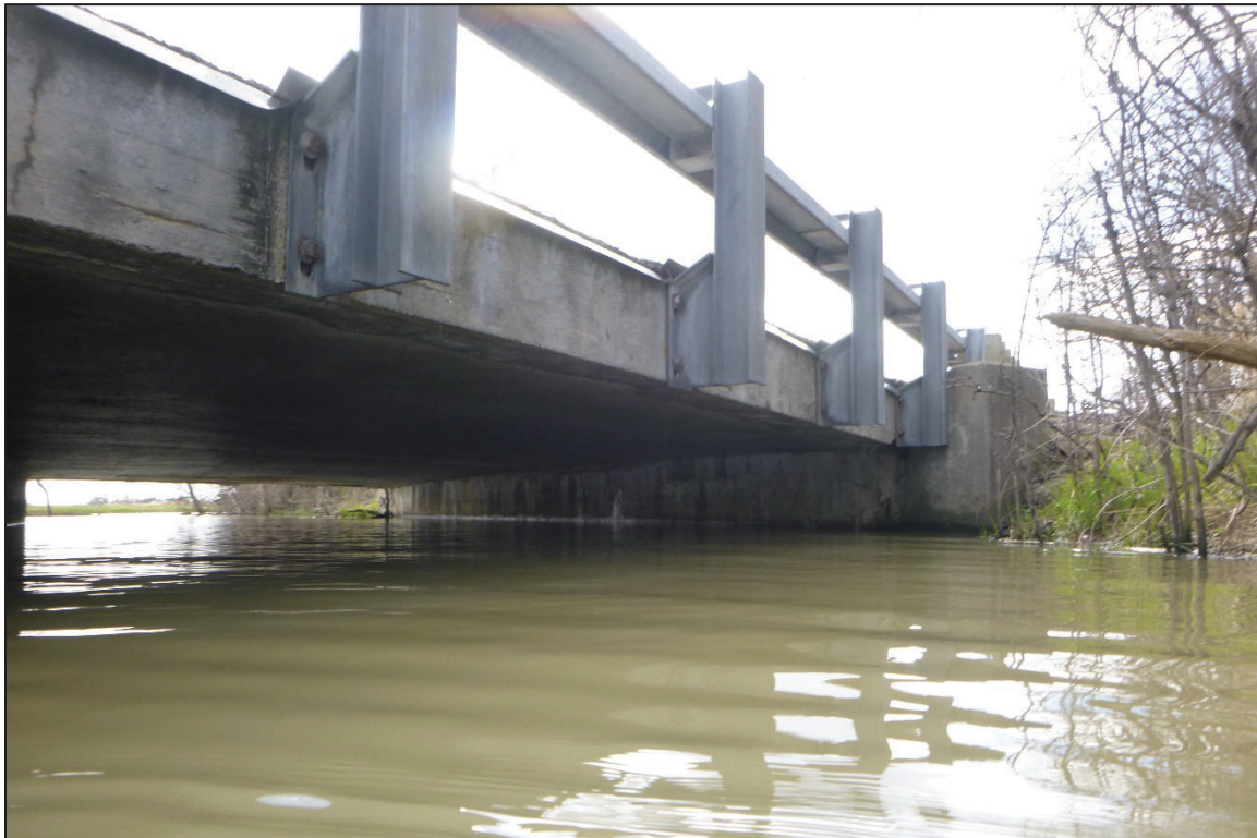
Photograph No. 4: View of the West Embankment at the Structure, Looking Southwest.
