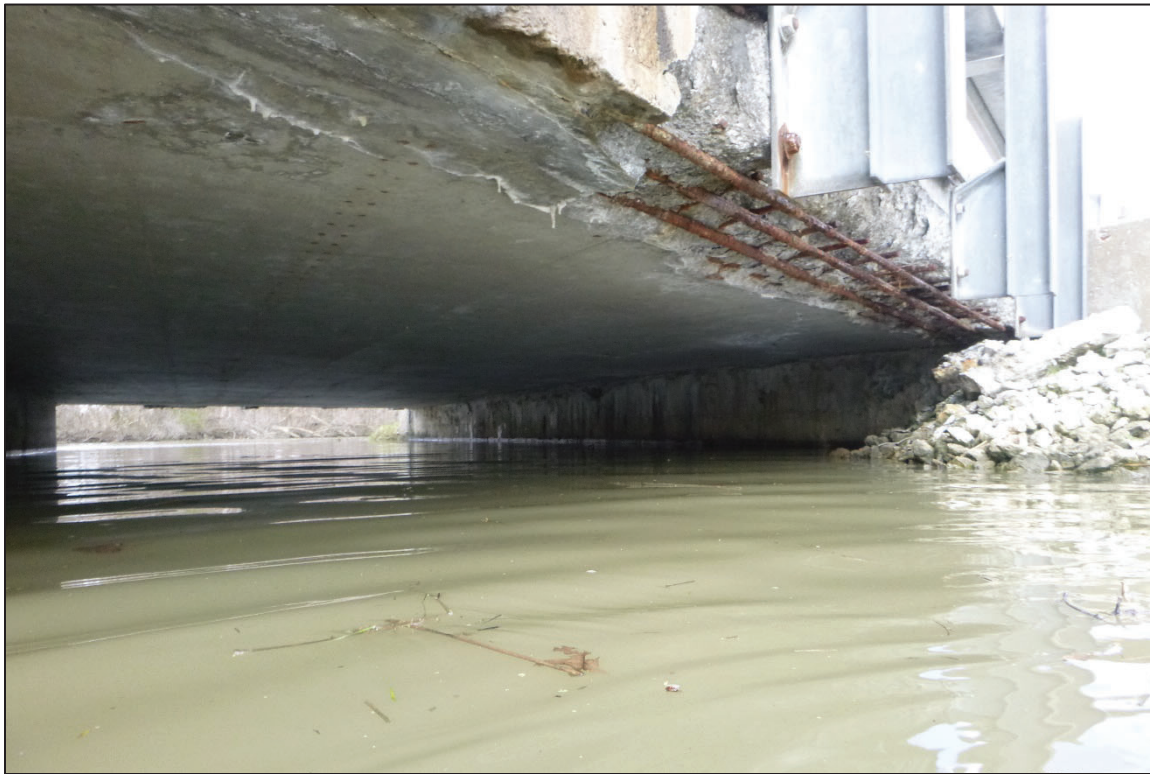
Photograph No. 7: View of the East Embankment at the Structure, Looking Northeast.
