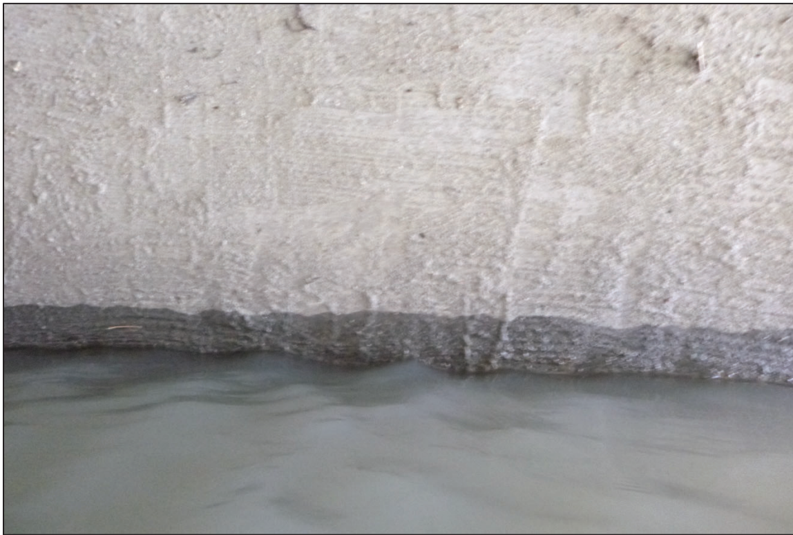
Photograph No. 18: View of the Typical Concrete Condition at the Waterline, Looking West.
