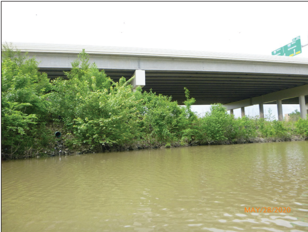
Photograph No. 6: View of the South Embankment Upstream of the Structure, Looking Southwest.
