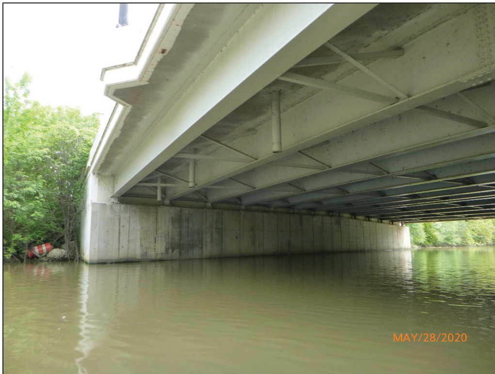
Photograph No. 4: View of the North Embankment at the Structure, Looking Northeast.
