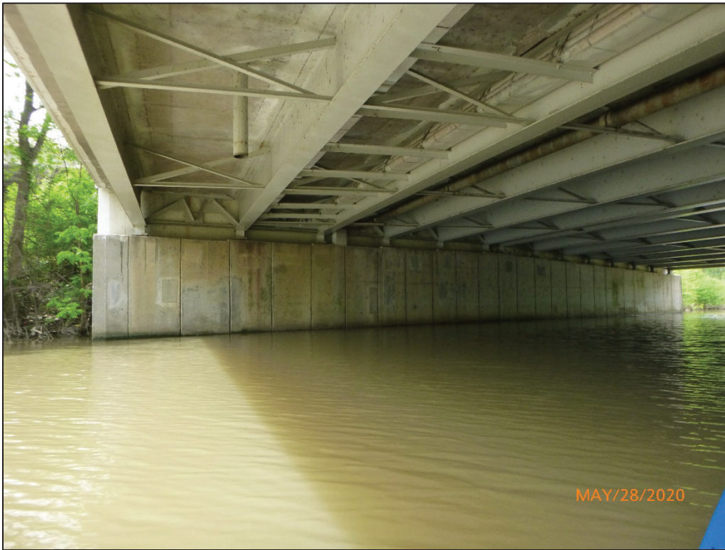
Photograph No. 7: View of the South Embankment at the Structure, Looking South.
