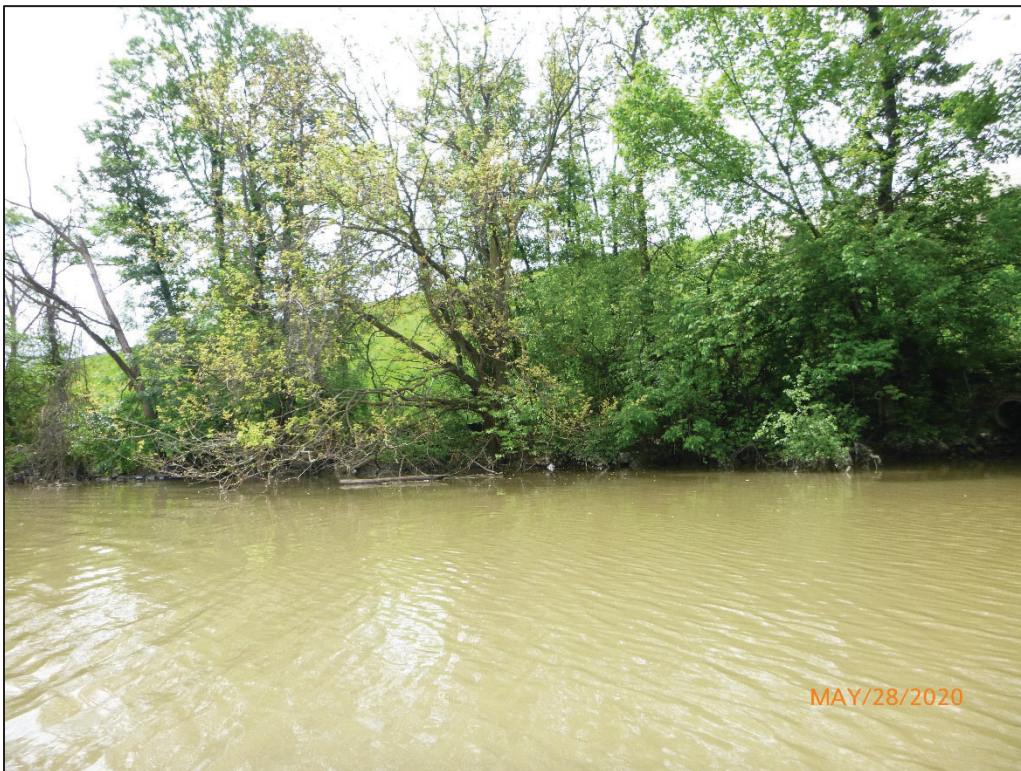
Photograph No. 8: View of the South Embankment Downstream of the Structure, Looking Southeast.
