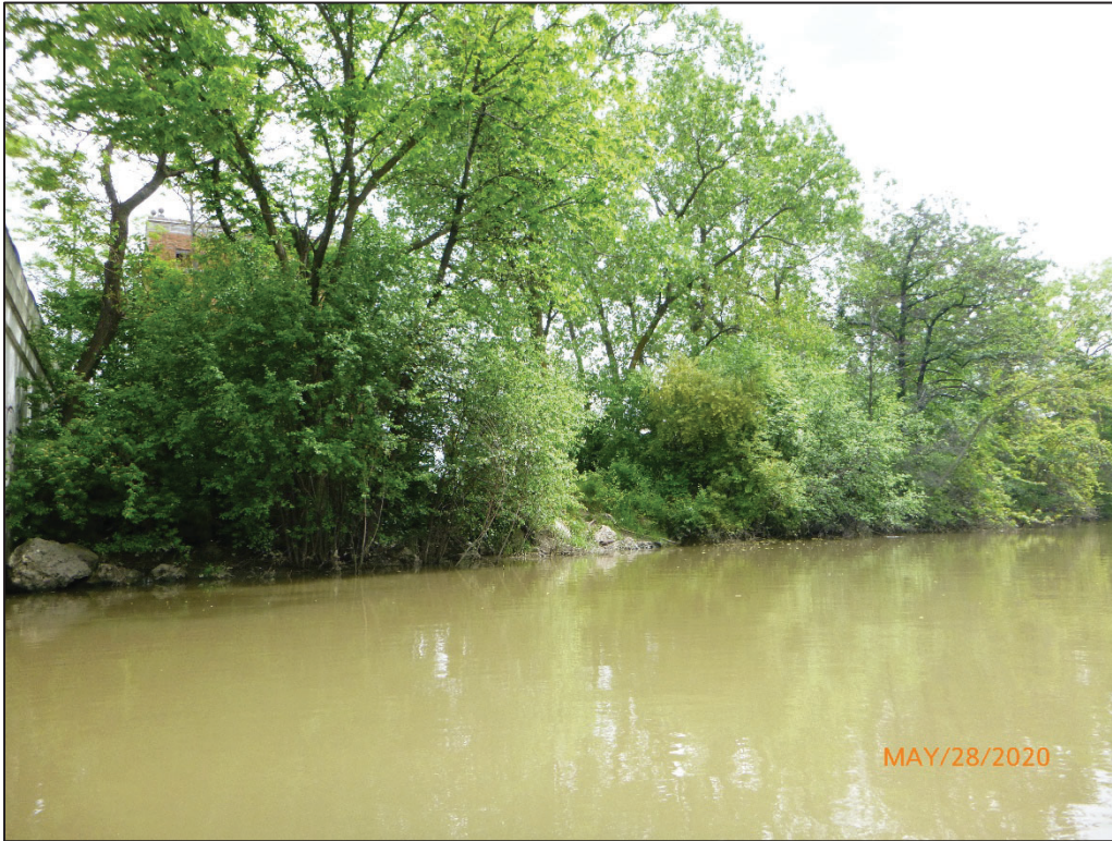
Photograph No. 5: View of the North Embankment Downstream of the Structure, Looking Northeast.
