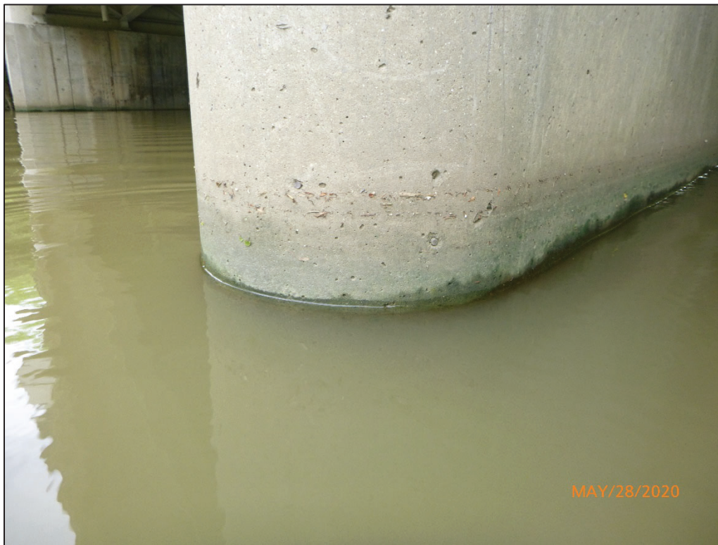
Photograph No. 11: View of the Typical Concrete Condition at the Waterline on the Upstream nose of Pier 1, Looking Northeast.
