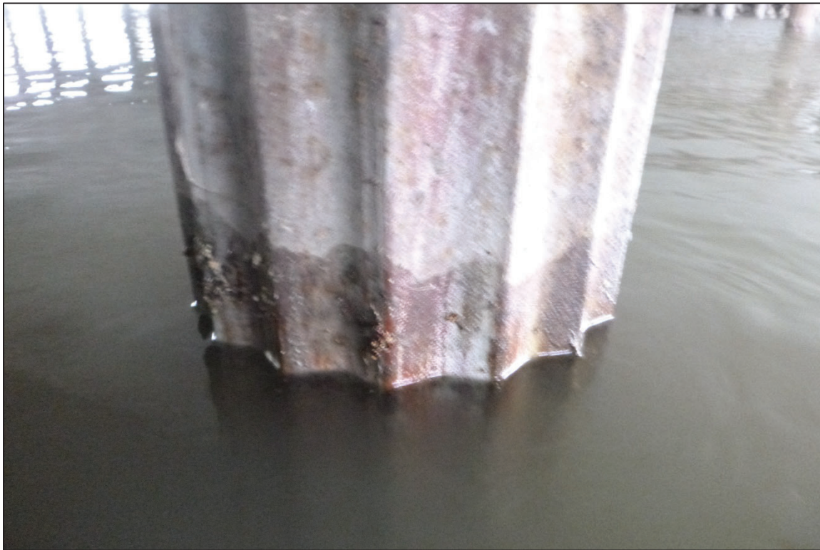
Photograph No. 27: View of the Typical Steel Condition at the Waterline, Looking Southwest.
