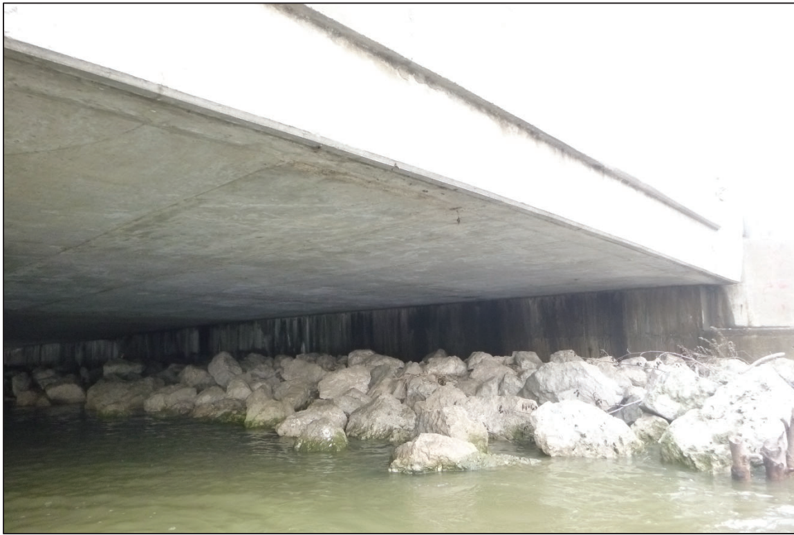
Photograph No. 5: View of the North Embankment at the Structure, Looking Northwest.
