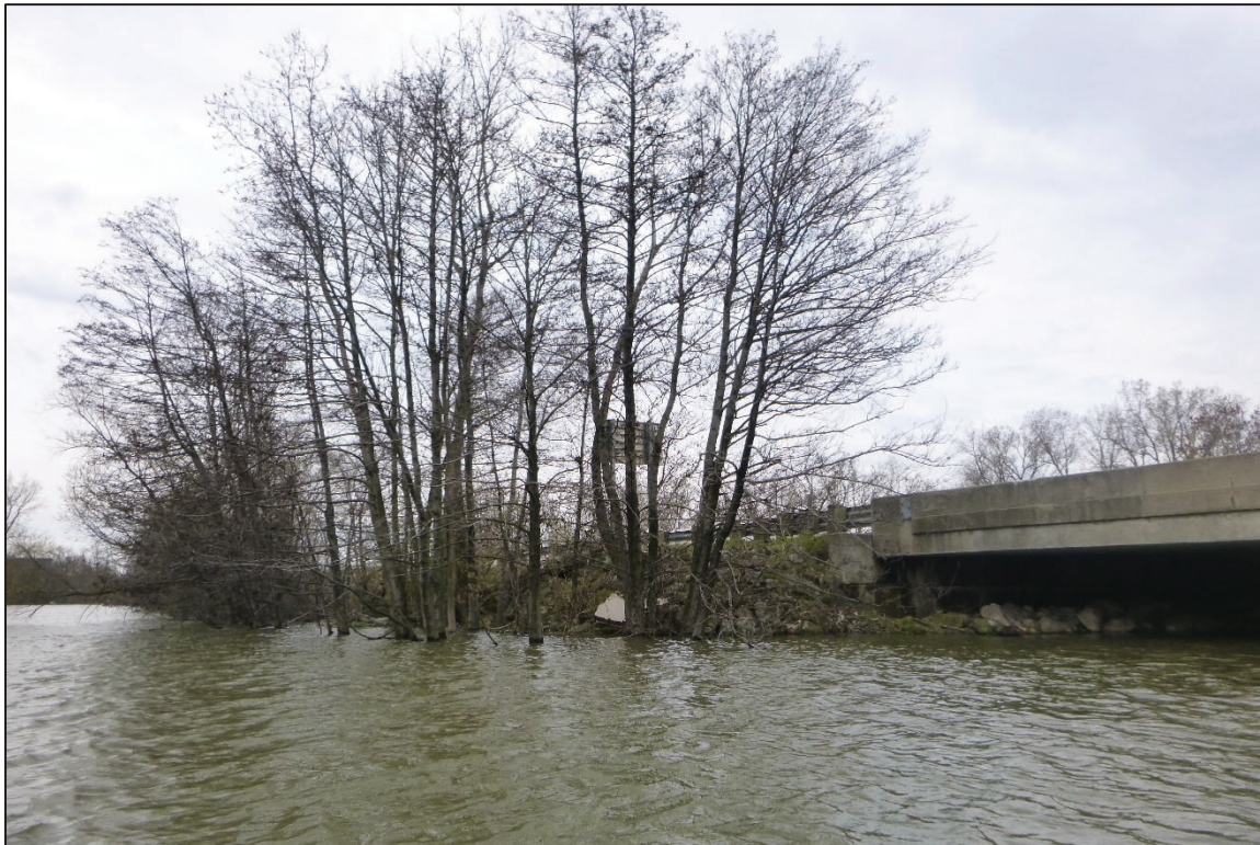
Photograph No. 10: View of the South Embankment Downstream of the Structure, Looking Southwest.
