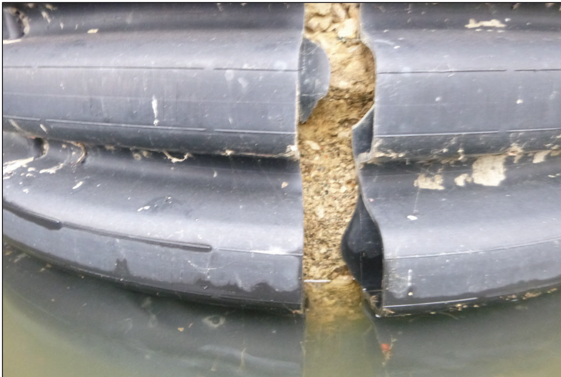
Photograph No. 28: View of the Typical Concrete Condition at the Waterline, Looking East.
