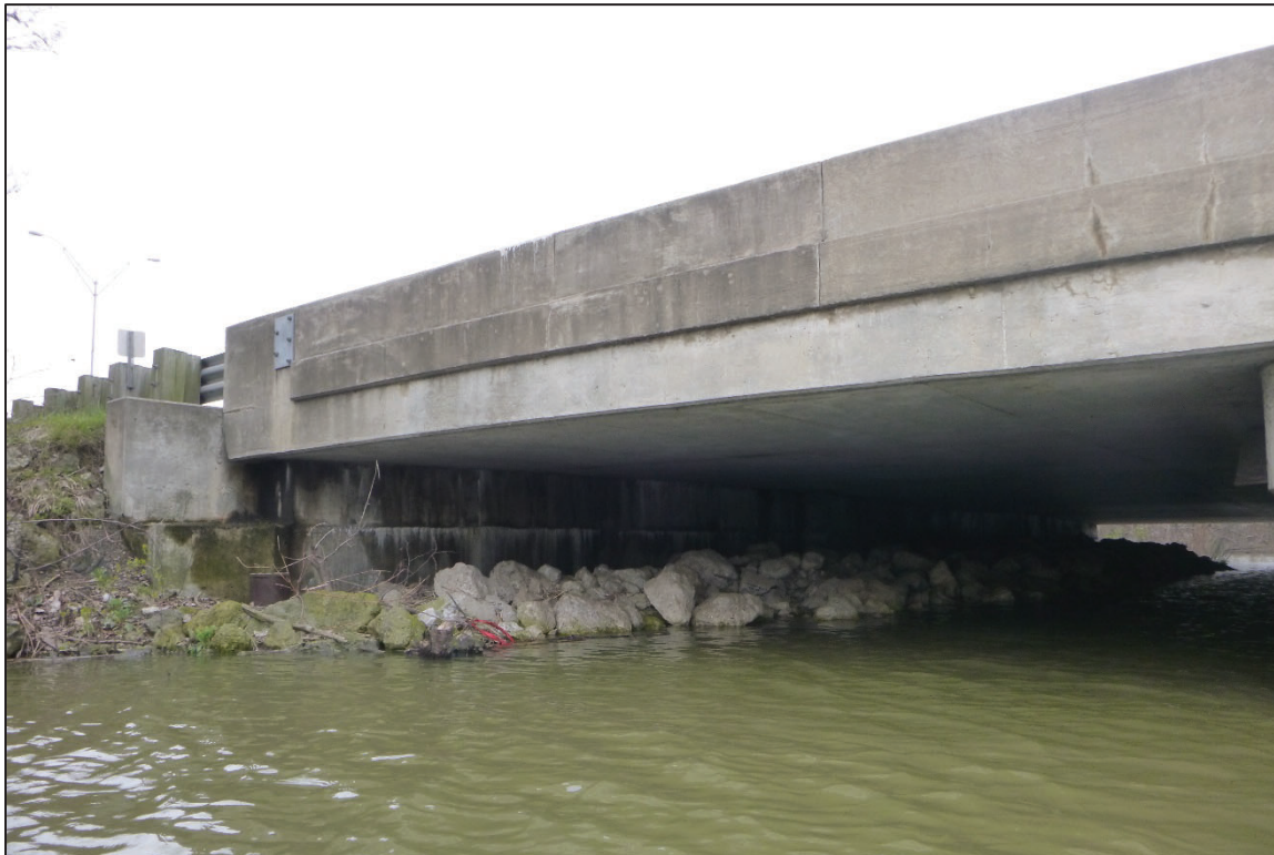
Photograph No. 8: View of the South Embankment at the Structure, Looking Southwest.
