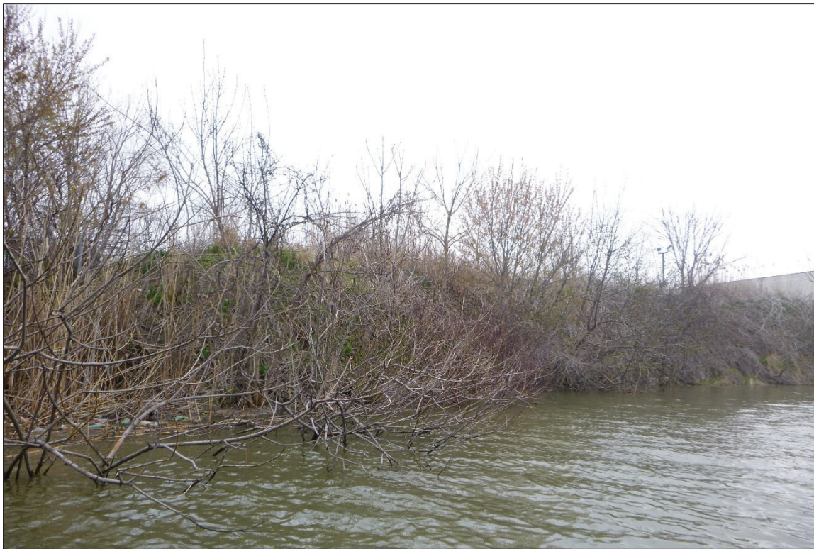
Photograph No. 6: View of the North Embankment Downstream of the Structure, Looking Northeast.
