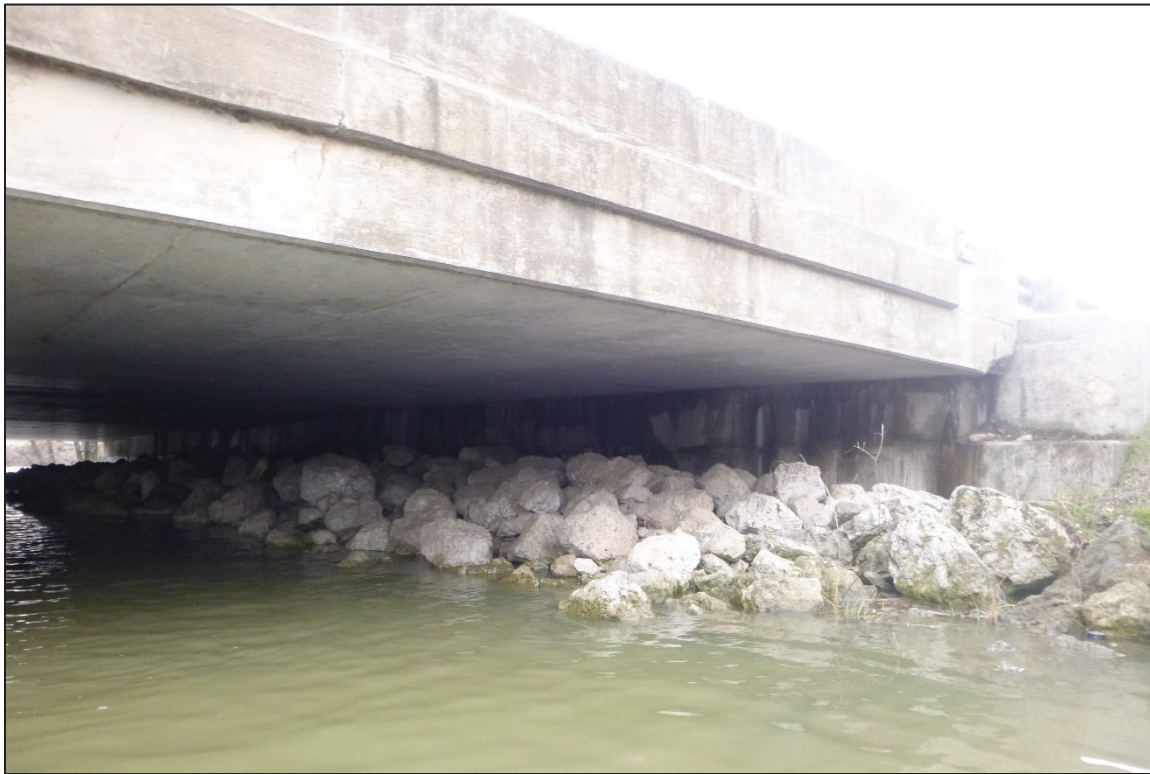
Photograph No. 9: View of the South Embankment at the Structure, Looking Southeast.
