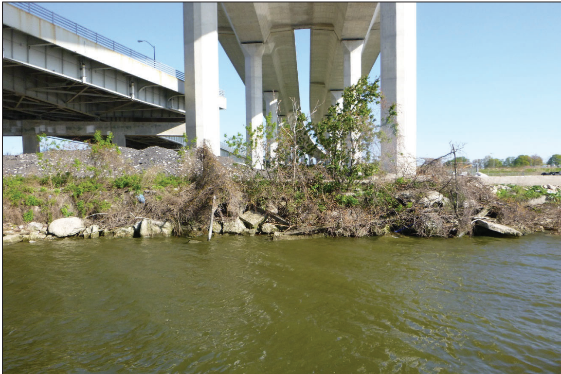
Photograph No. 4: View of the Northwest Embankment at the Structure, Looking Northwest.
