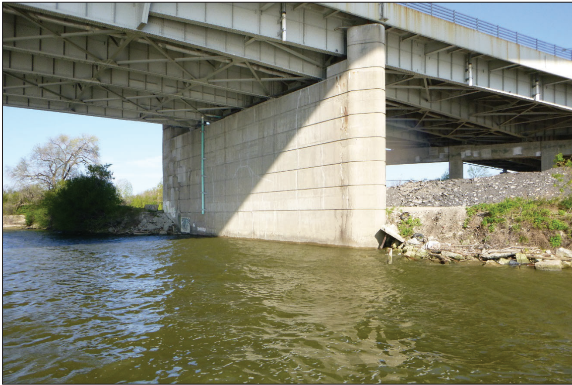
Photograph No. 3: View of the Northwest Embankment Upstream of the Structure, Looking West.
