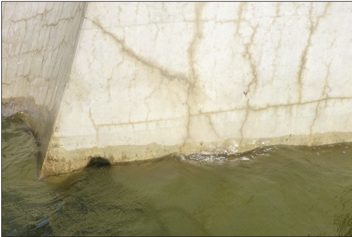
Photograph No. 11: View of the Typical Concrete Condition at the Waterline, Looking North.
