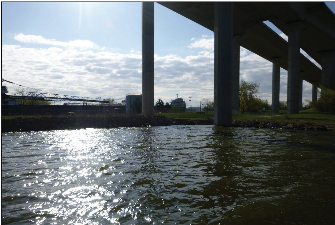
Photograph No. 8: View of the Southeast Embankment Downstream of the Structure, Looking Southeast.
