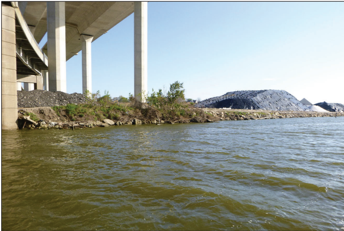
Photograph No. 5: View of the Northwest Embankment Downstream of the Structure, Looking North.
