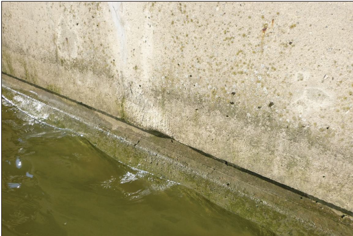
Photograph No. 18: View of the Typical Concrete Condition at the Waterline, Looking Southwest.
