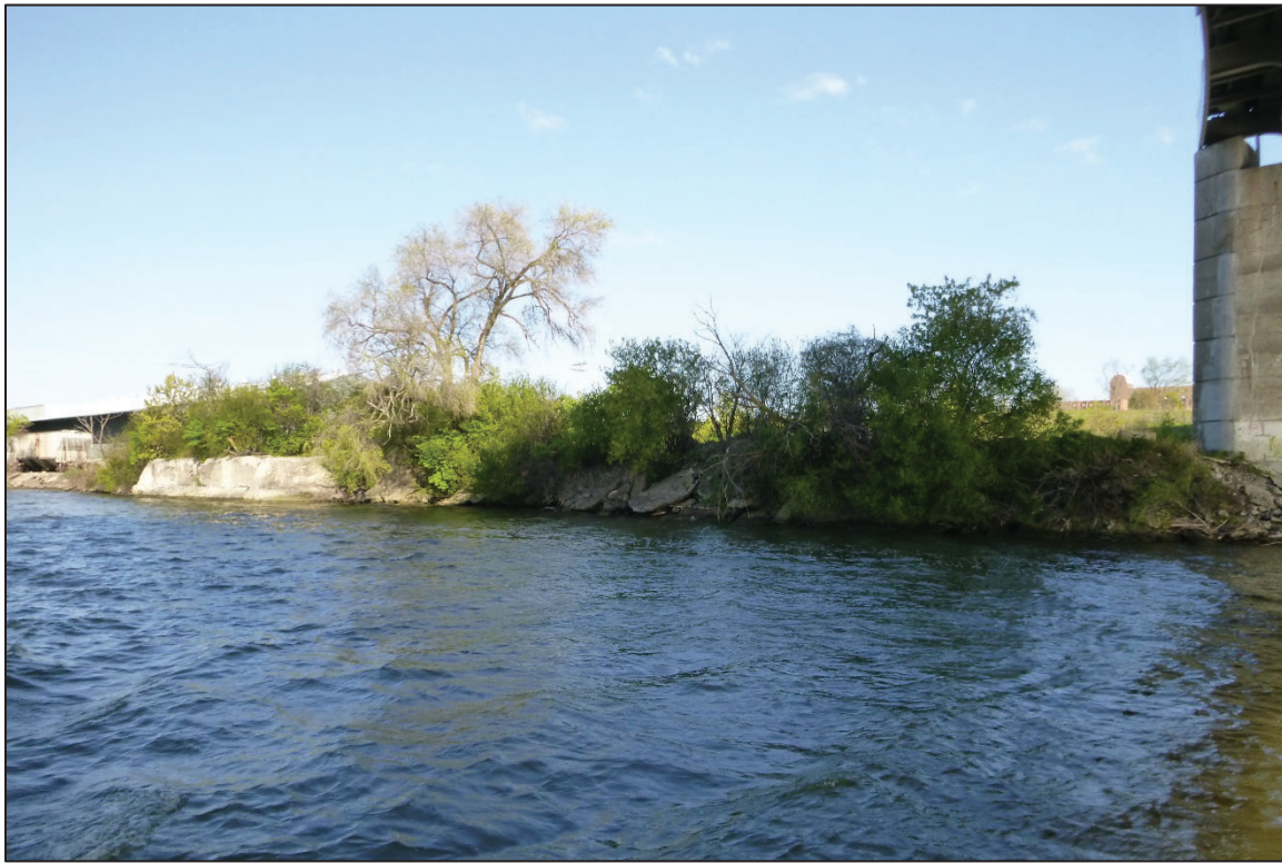
Photograph No. 3: View of the Northwest Embankment Upstream of the Structure, Looking Northwest.
