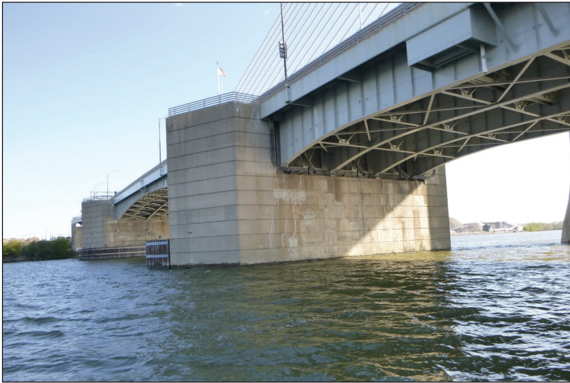
Photograph No. 15: View of the South Face of Bascule Pier 4, Looking North.
