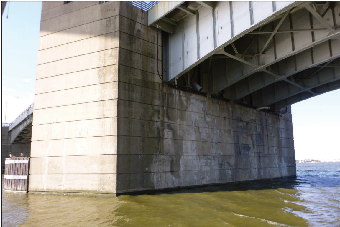
Photograph No. 16: View of the North Face of Bascule Pier 5, Looking South.
