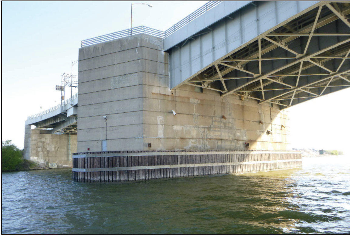
Photograph No. 17: View of the South Face of Bascule Pier 5, Looking North.
