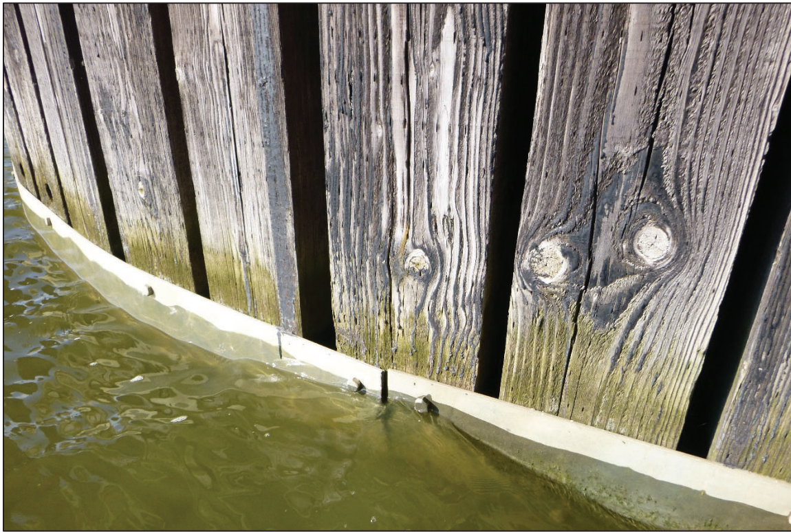
Photograph No. 19: View of the Typical Fender Condition at the Waterline, Looking Southwest.
