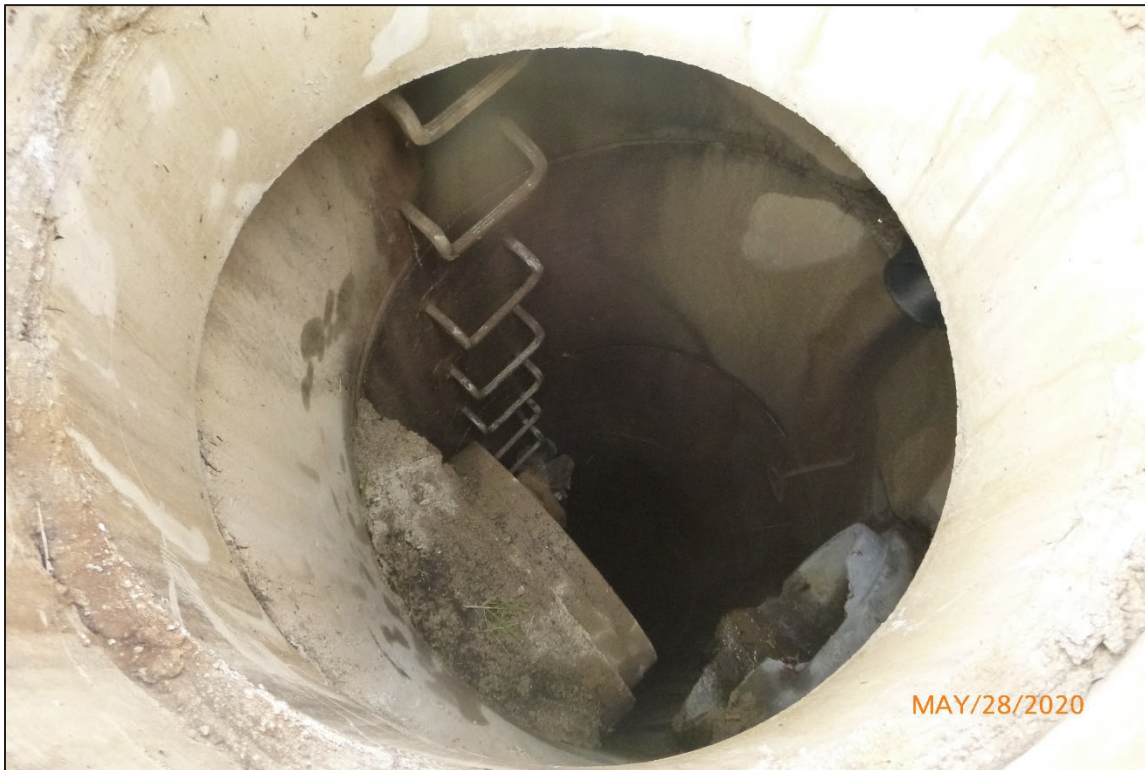
Photograph No. 2: Overall View of Manhole for Structure No. 4808428 (LUC-475-1503), Looking East.
