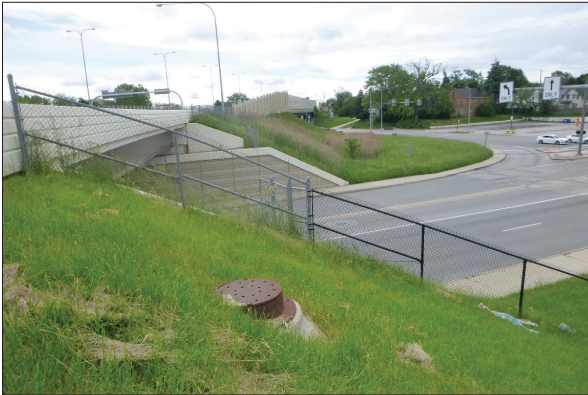
Photograph No. 1: Overall View of Access Location for Structure No. 4808479 (LUC-475-1538), Looking East.
