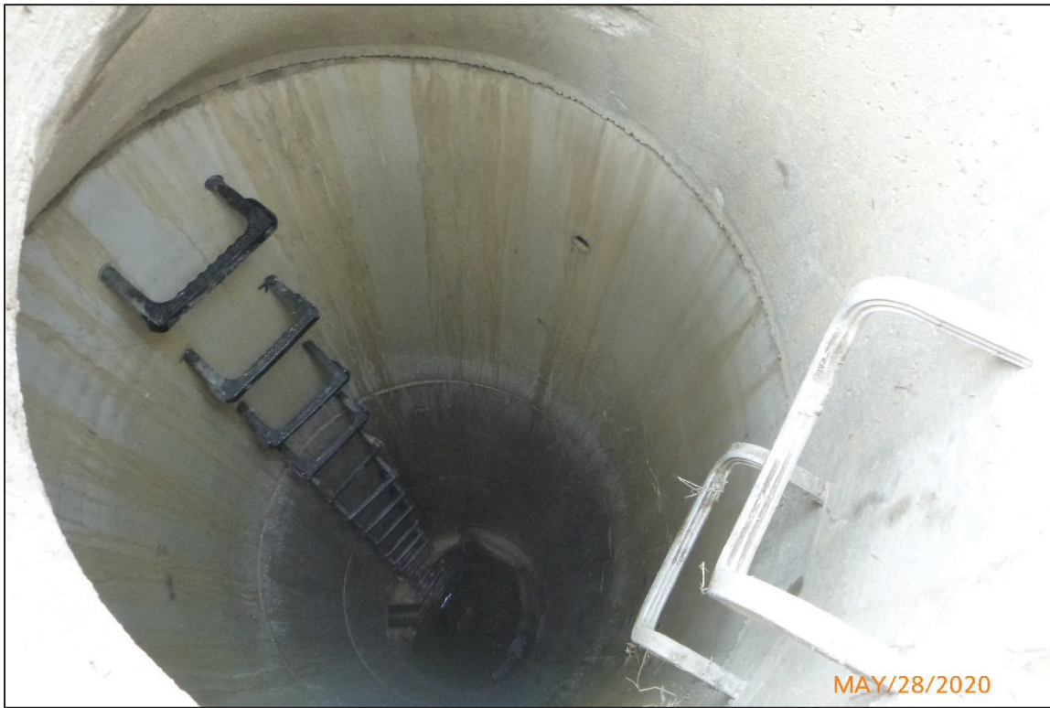
Photograph No. 2: Overall View of Manhole for Structure No. 4808479 (LUC-475-1538), Looking East.
