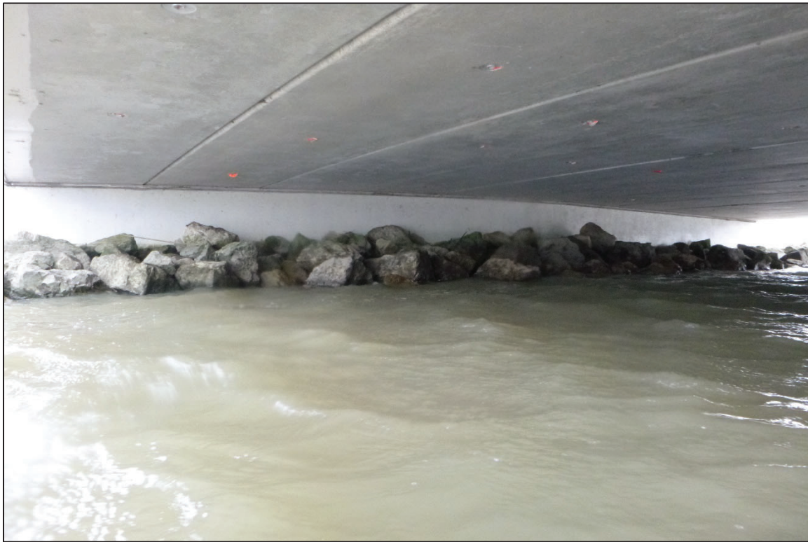
Photograph No. 7: View of the South Embankment at the Structure, Looking South.
