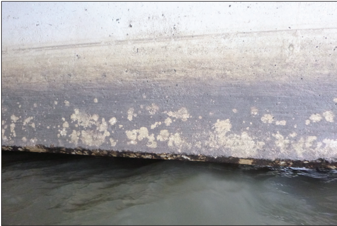
Photograph No. 13: View of the Typical Concrete Condition at the Waterline, Looking South.
