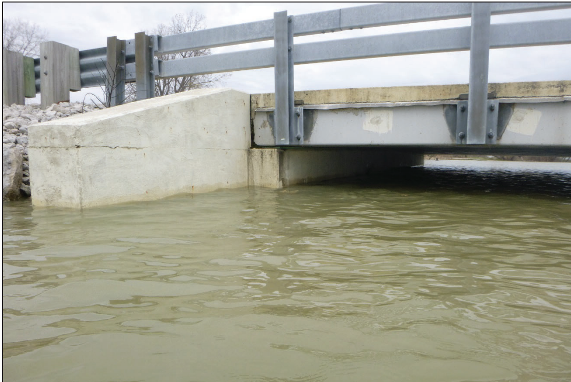
Photograph No. 8: View of the West Embankment at the Structure, Looking Northwest.
