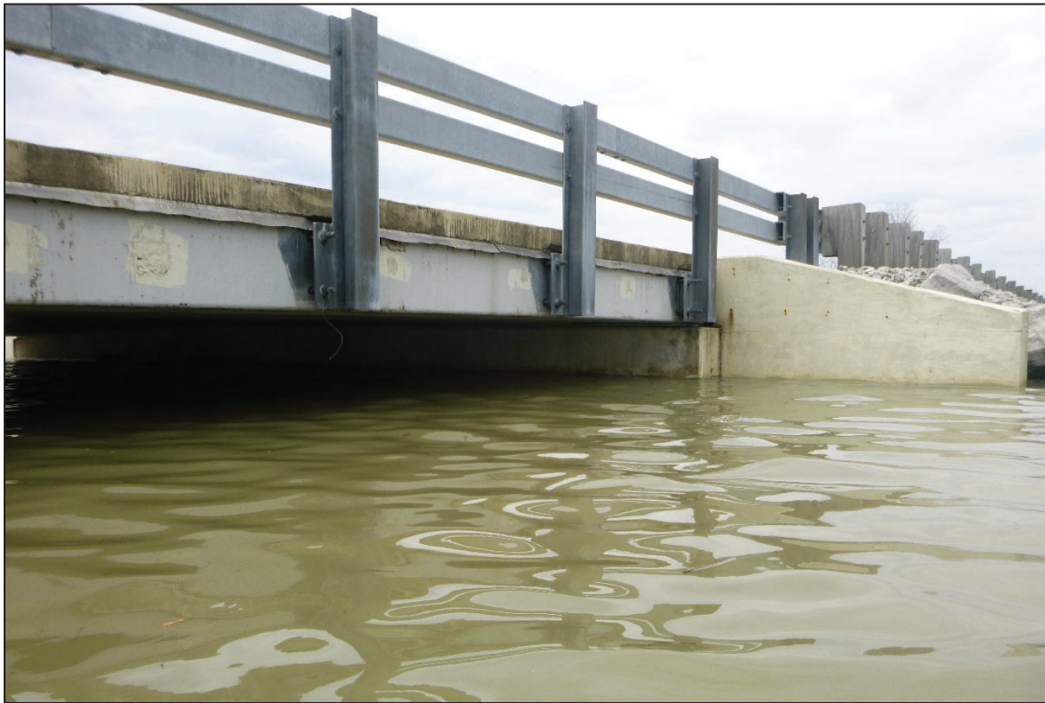
Photograph No. 9: View of the West Embankment at the Structure, Looking Southwest.
