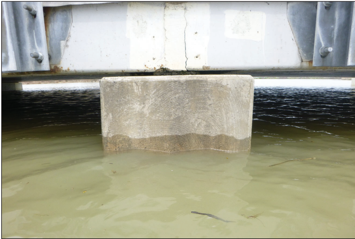
Photograph No. 15: View of the Typical Concrete Condition at the Waterline, Looking North.
