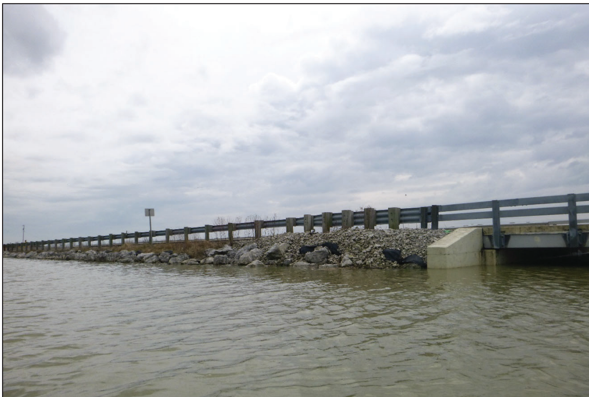
Photograph No. 6: View of the East Embankment Downstream of the Structure, Looking Southeast.
