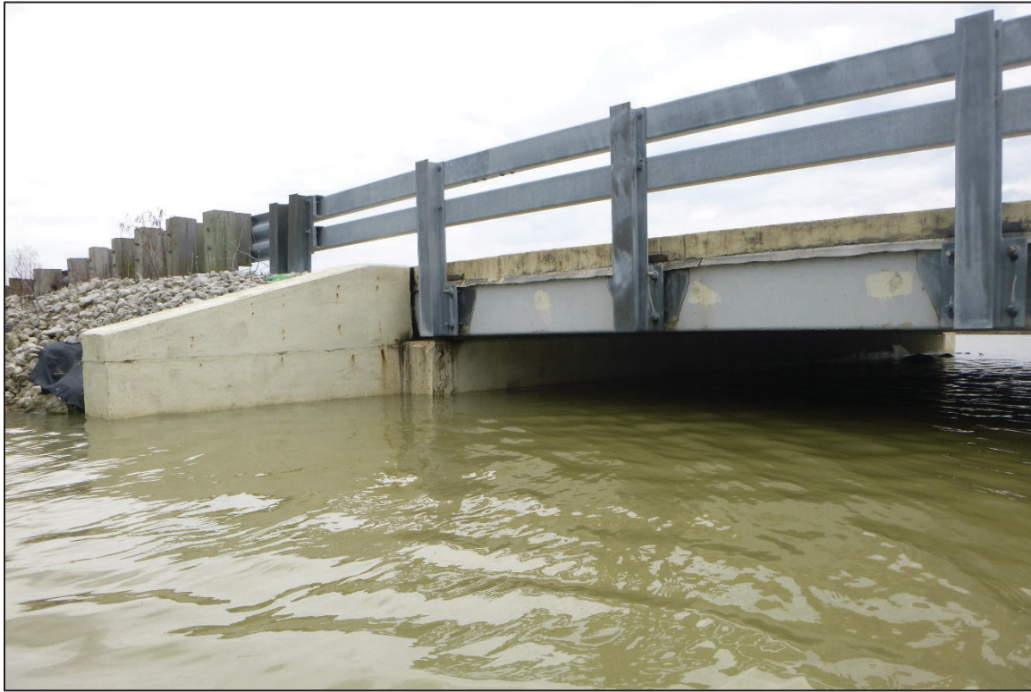
Photograph No. 3: View of the East Embankment Upstream of the Structure, Looking Southeast.
