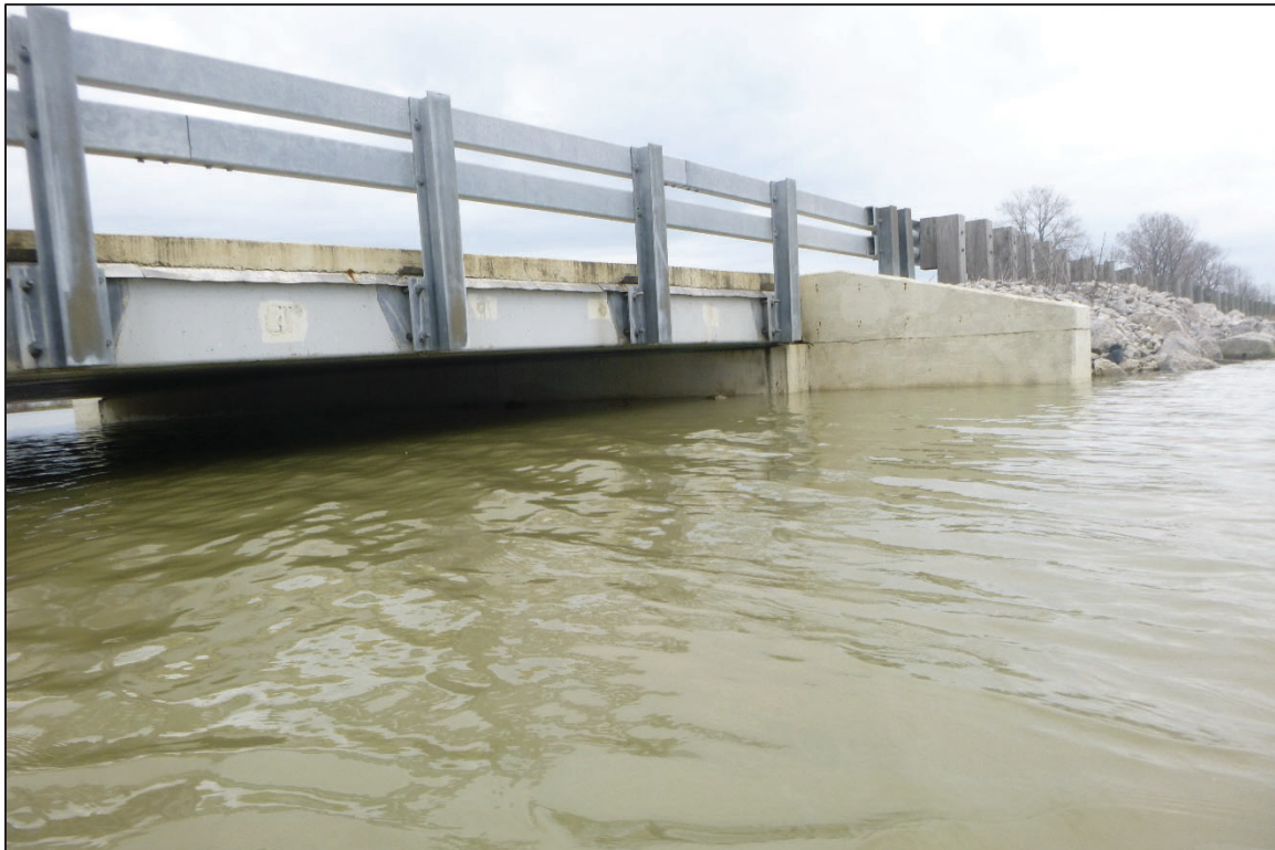
Photograph No. 4: View of the East Embankment at the Structure, Looking Northeast.
