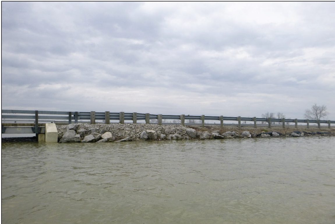
Photograph No. 10: View of the West Embankment Downstream of the Structure, Looking Southwest.
