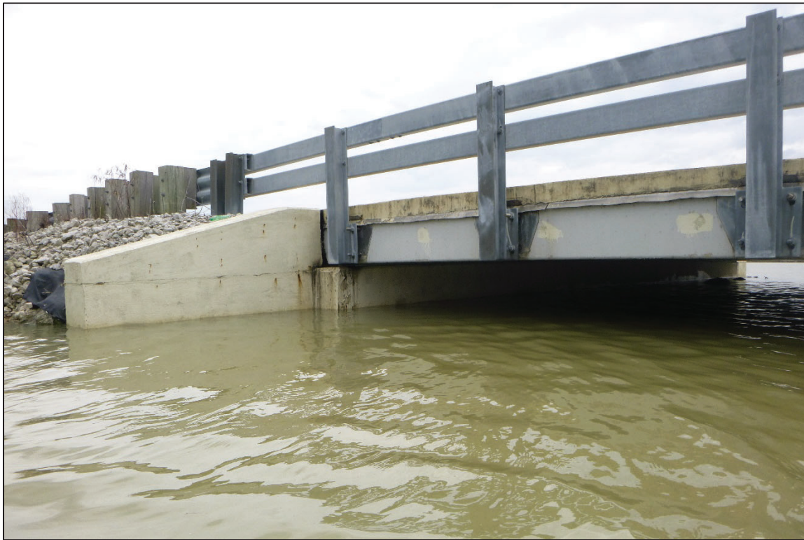
Photograph No. 5: View of the East Embankment at the Structure, Looking Southeast.
