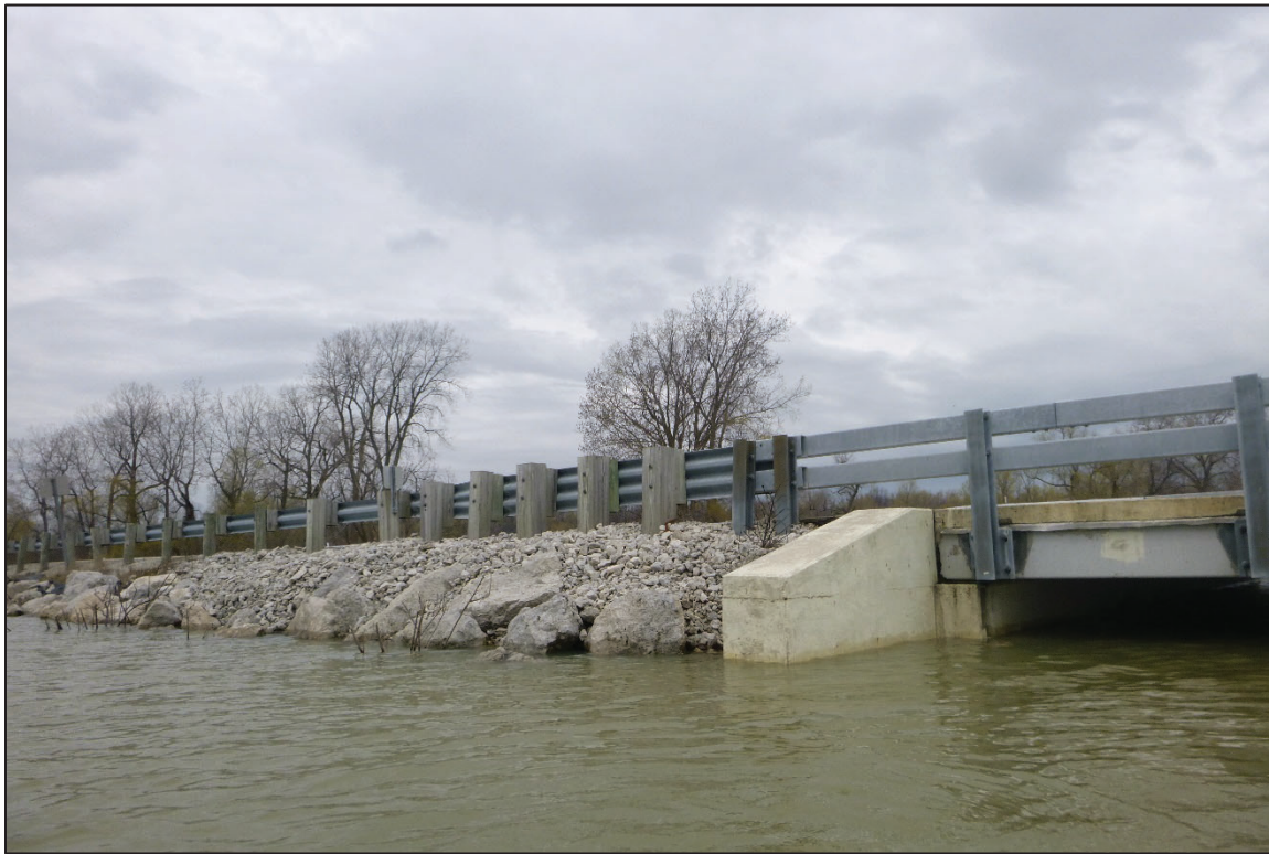
Photograph No. 7: View of the West Embankment Upstream of the Structure, Looking Northwest.
