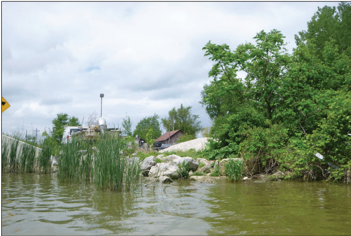
Photograph No. 5: View of the North Embankment Downstream of the Structure, Looking North.
