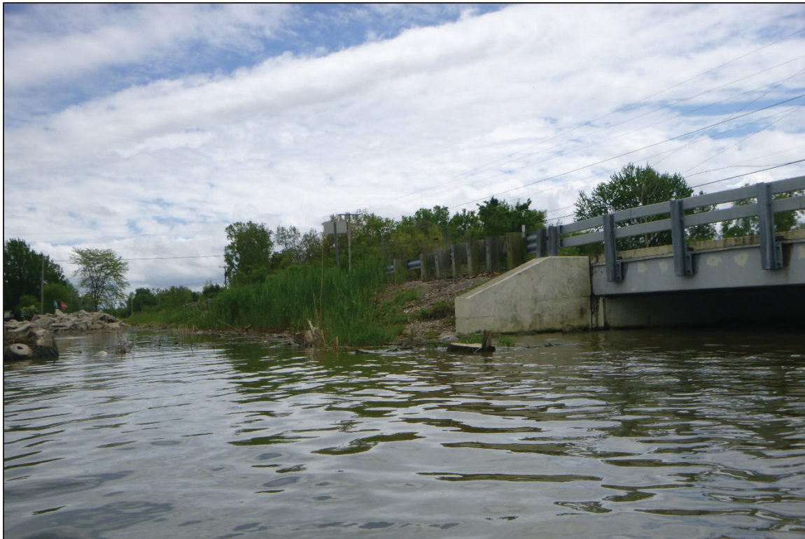
Photograph No. 8: View of the South Embankment Downstream of the Structure, Looking Southwest.
