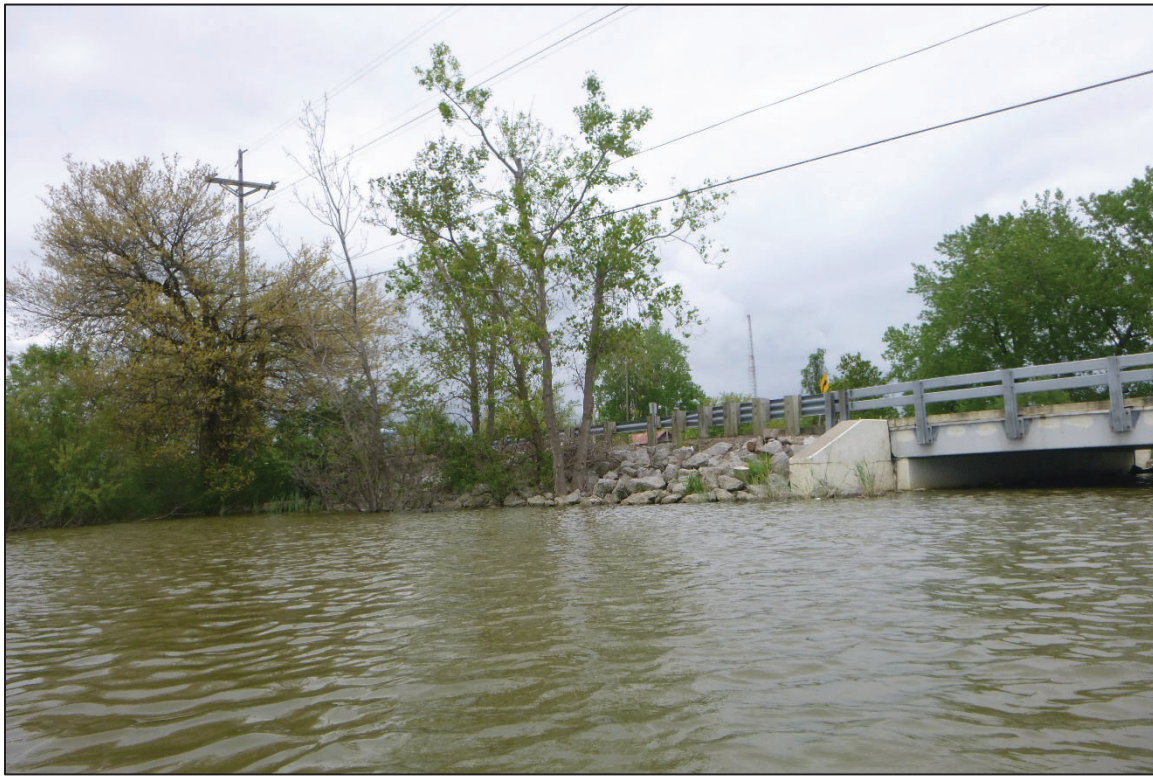
Photograph No. 3: View of the North Embankment Upstream of the Structure, Looking Northeast.
