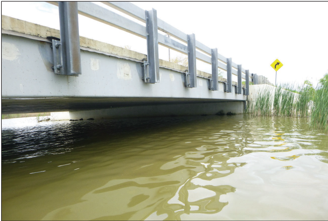
Photograph No. 7: View of the South Embankment at the Structure, Looking Northwest.
