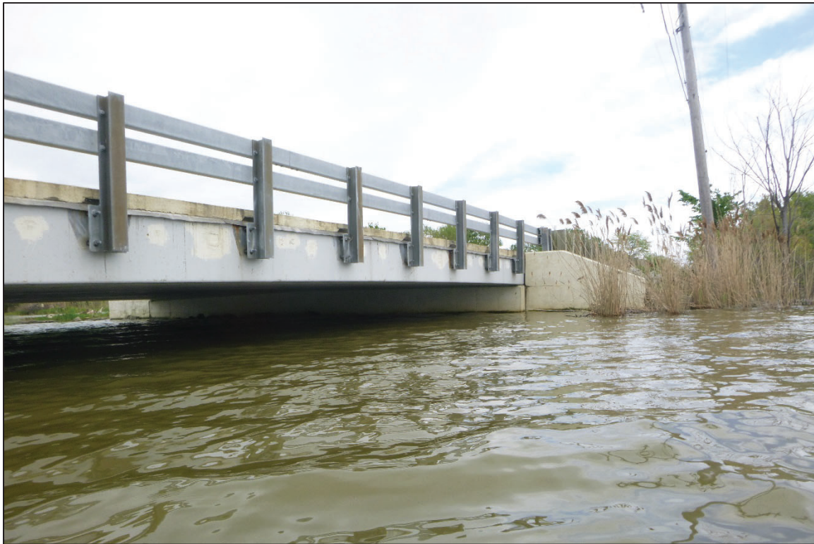
Photograph No. 4: View of the North Embankment at the Structure, Looking Southeast.
