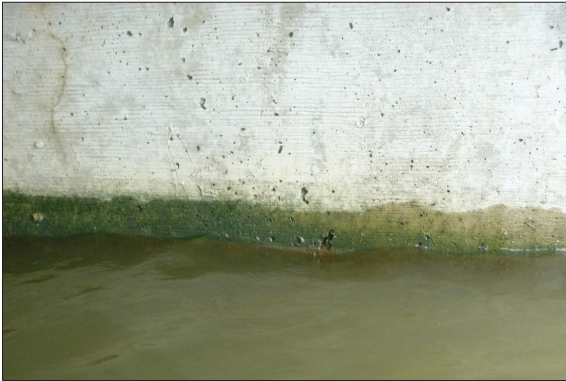
Photograph No. 19: View of the Typical Concrete Condition at the Waterline, Looking North.
