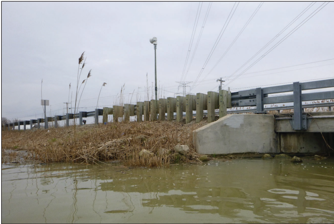
Photograph No. 9: View of the East Embankment Downstream of the Structure, Looking South.
