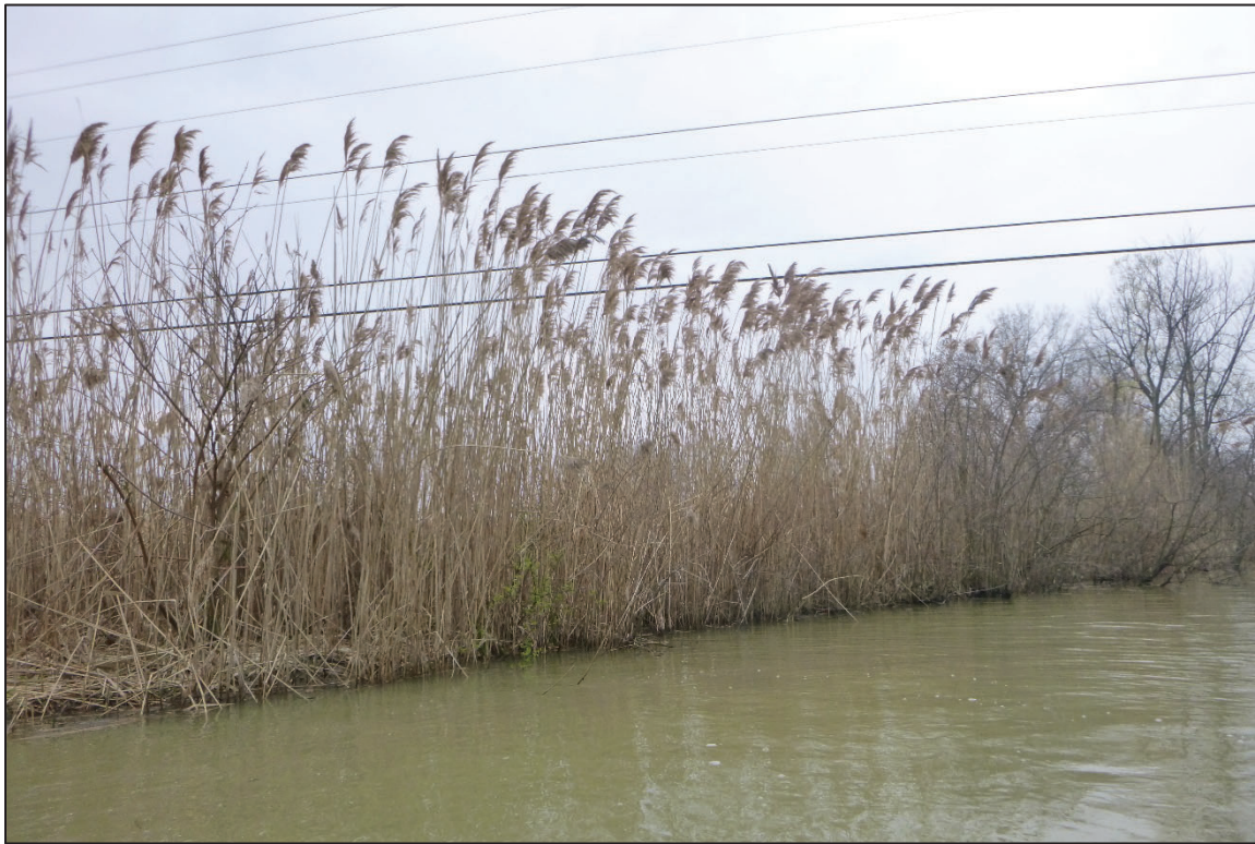
Photograph No. 7: View of the East Embankment Upstream of the Structure, Looking South.
