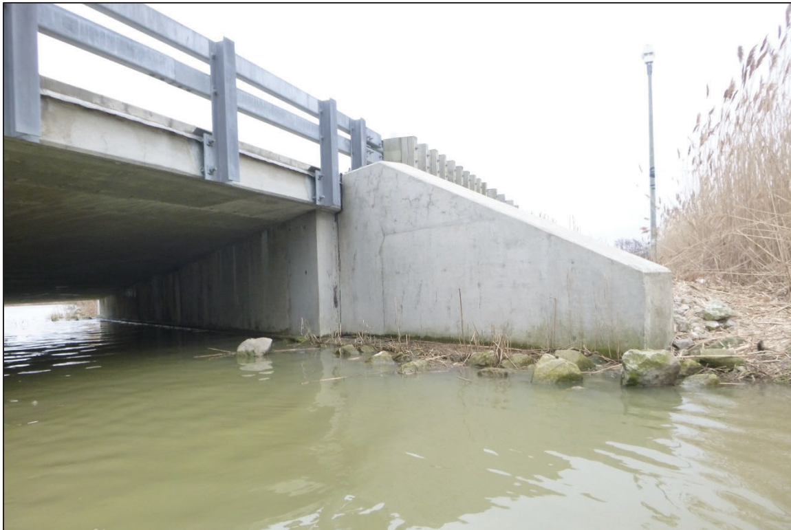
Photograph No. 8: View of the East Embankment at the Structure, Looking East.
