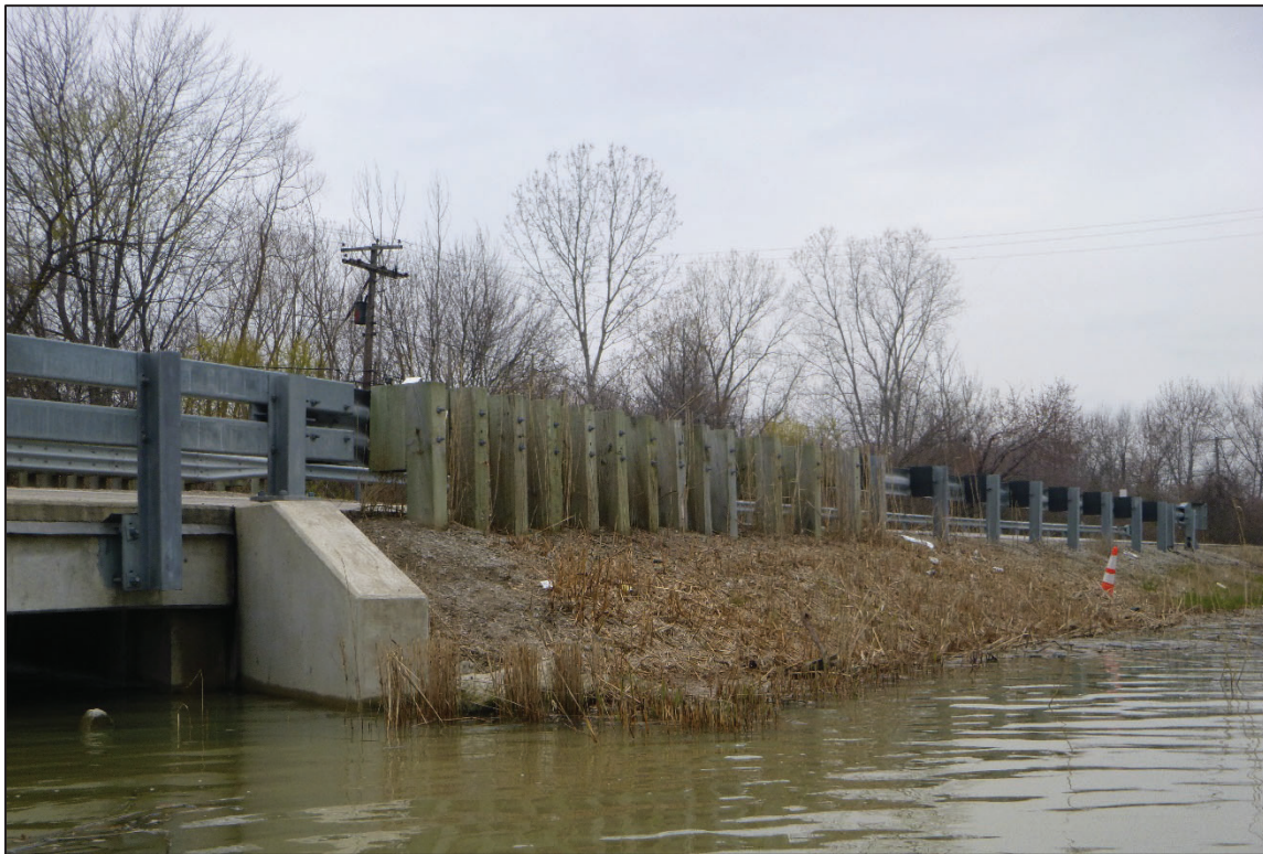
Photograph No. 6: View of the West Embankment Downstream of the Structure, Looking West.
