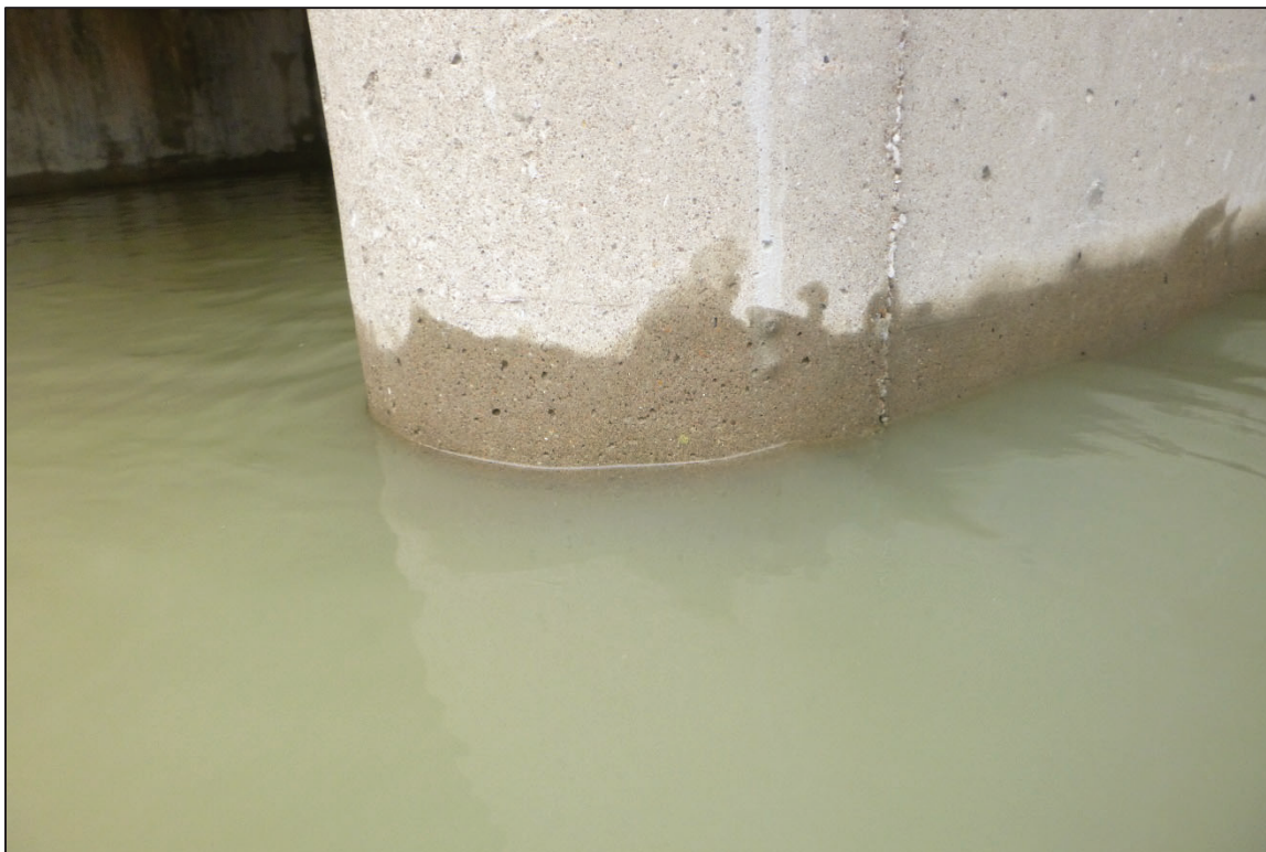
Photograph No. 14: View of the Typical Concrete Condition at the Waterline, Looking North.
