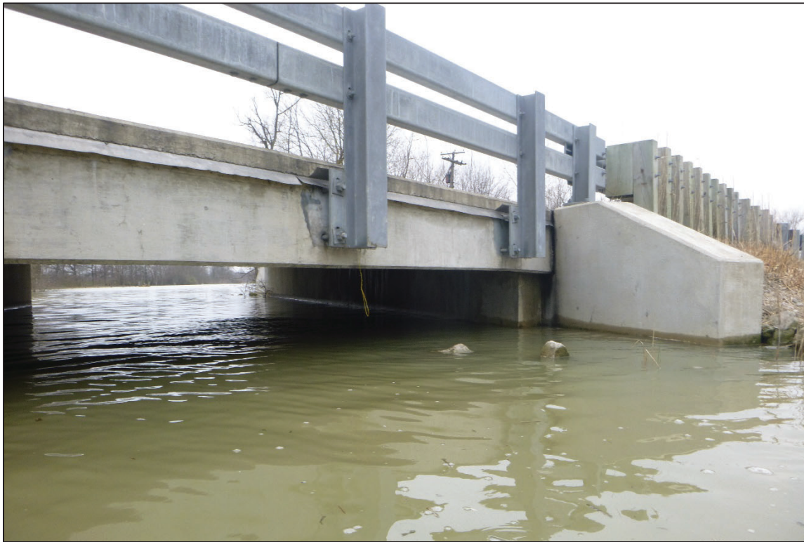
Photograph No. 5: View of the West Embankment at the Structure, Looking North.
