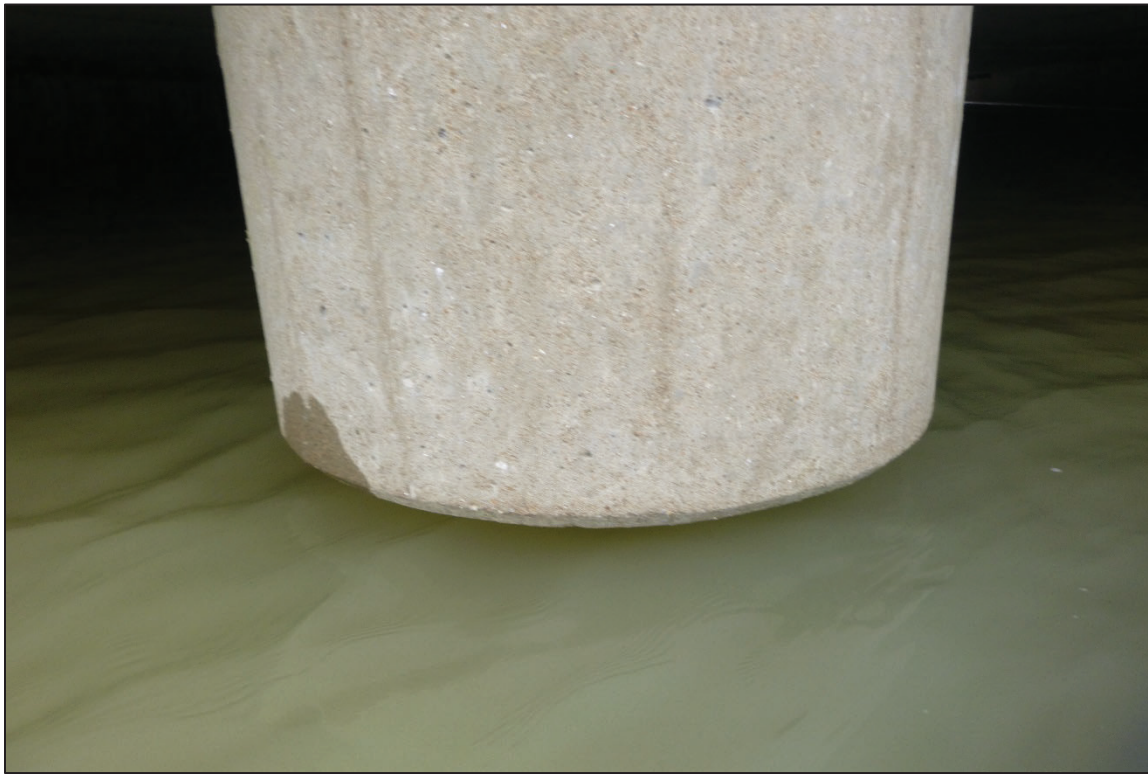
Photograph No. 13: View of the Typical Concrete Condition at the Waterline, Looking Southwest.
