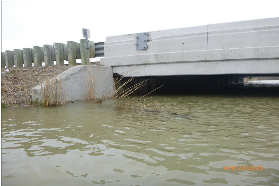
Photograph No. 4: View of the West Embankment at the Structure, Looking North.
