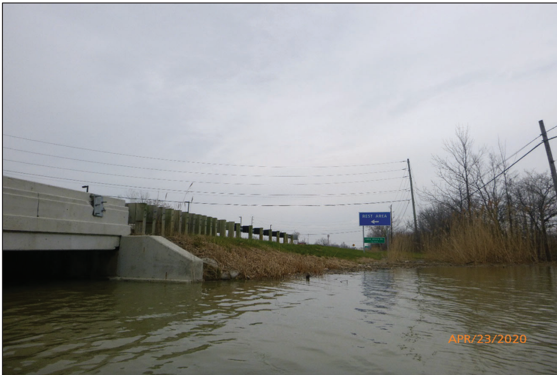
Photograph No. 6: View of the East Embankment Upstream of the Structure, Looking South.
