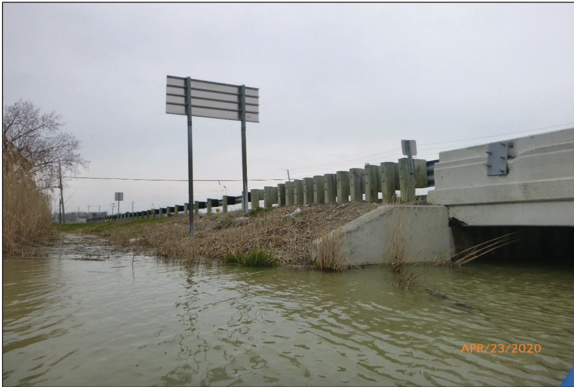
Photograph No. 3: View of the West Embankment Upstream of the Structure, Looking North.
