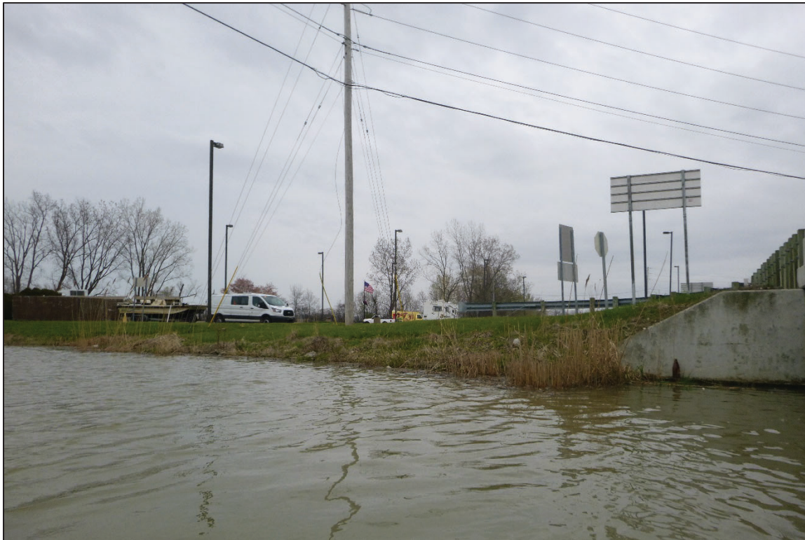
Photograph No. 8: View of the East Embankment Downstream of the Structure, Looking East.
