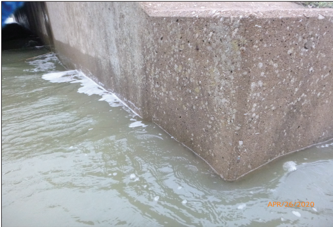
Photograph No. 11: View of the Typical Concrete Condition at the Waterline on the South Corner of Abutment 2, Looking Northeast.
