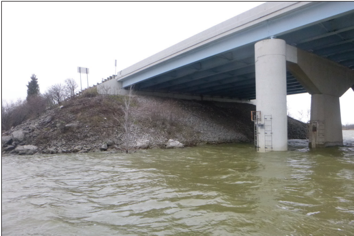
Photograph No. 4: View of the West Embankment at the Structure, Looking Northwest.
