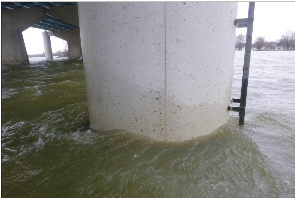
Photograph No. 20: View of the Typical Concrete Condition of the Caisson at the Waterline.
