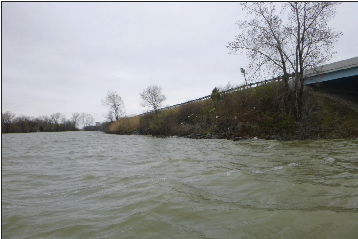
Photograph No. 8: View of the East Embankment Downstream of the Structure, Looking South.
