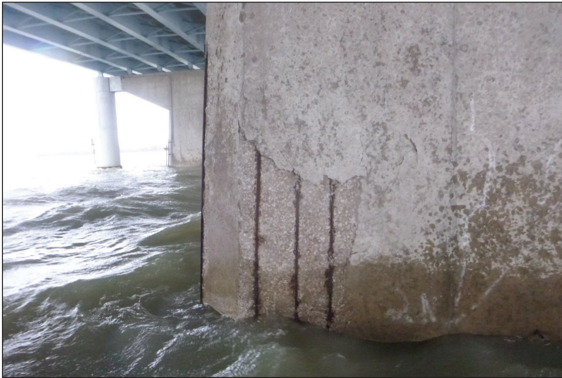
Photograph No. 13: View of the Spall at the Upstream Nose of Pier 2.
