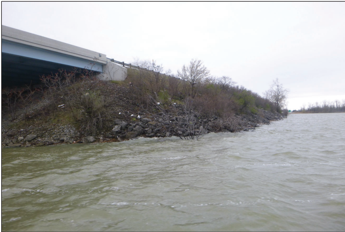
Photograph No. 5: View of the West Embankment Downstream of the Structure, Looking West.
