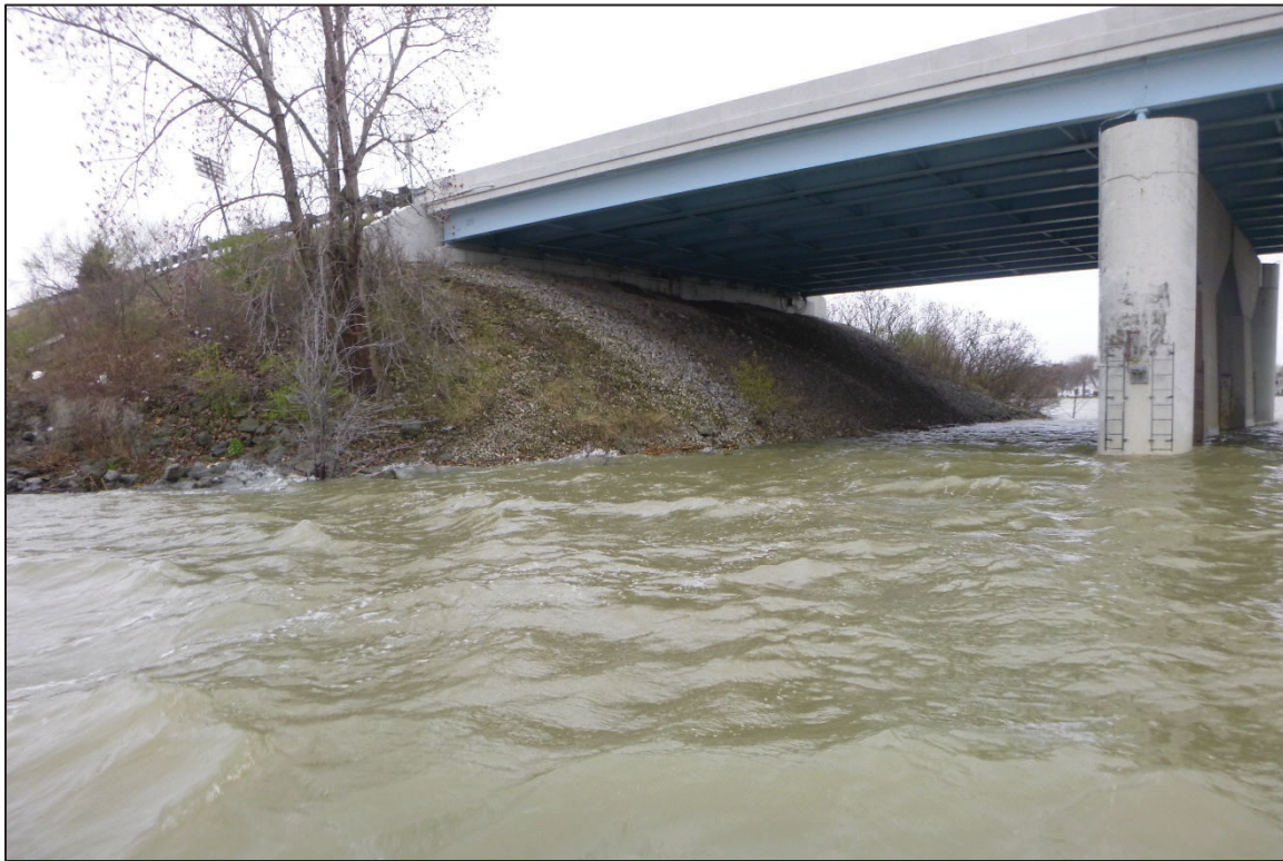
Photograph No. 7: View of the East Embankment at the Structure, Looking South.
