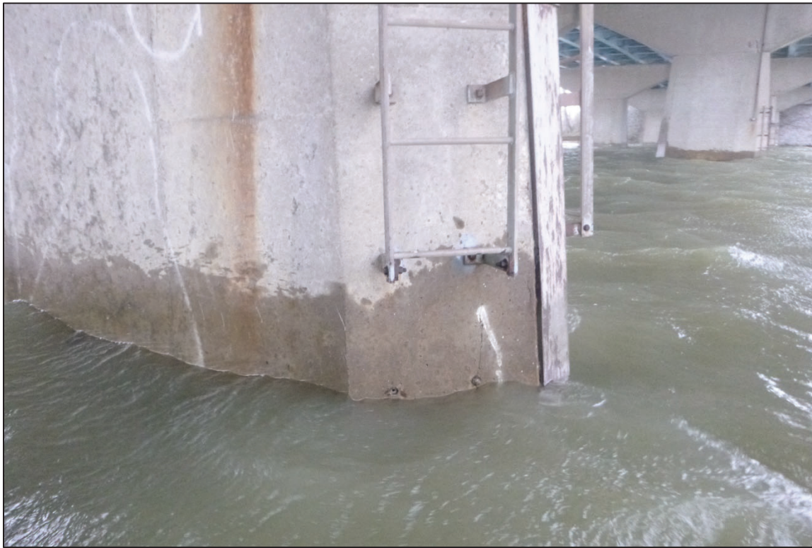
Photograph No. 21: View of the Typical Concrete Condition at the Pier at the Waterline.
