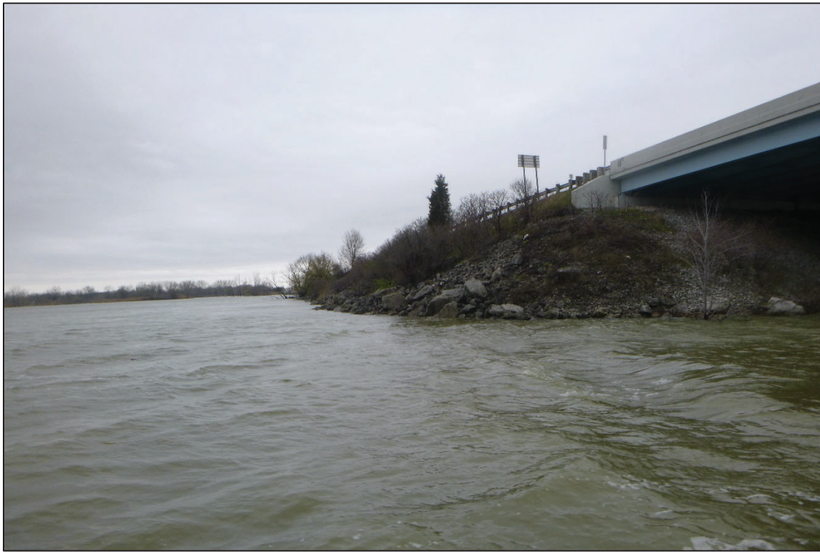
Photograph No. 3: View of the West Embankment Upstream of the Structure, Looking West.
