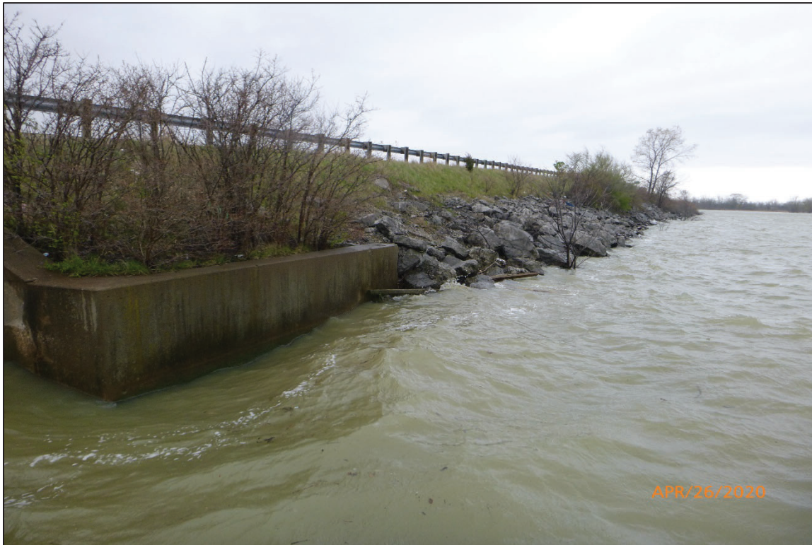
Photograph No. 4: View of the West Embankment Downstream of the Structure, Looking Southwest.
