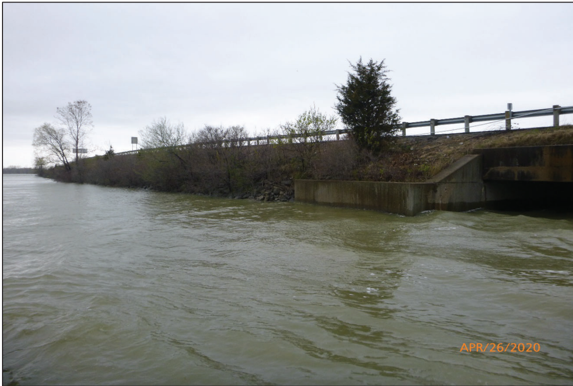
Photograph No. 3: View of the West Embankment Upstream of the Structure, Looking Northwest.
