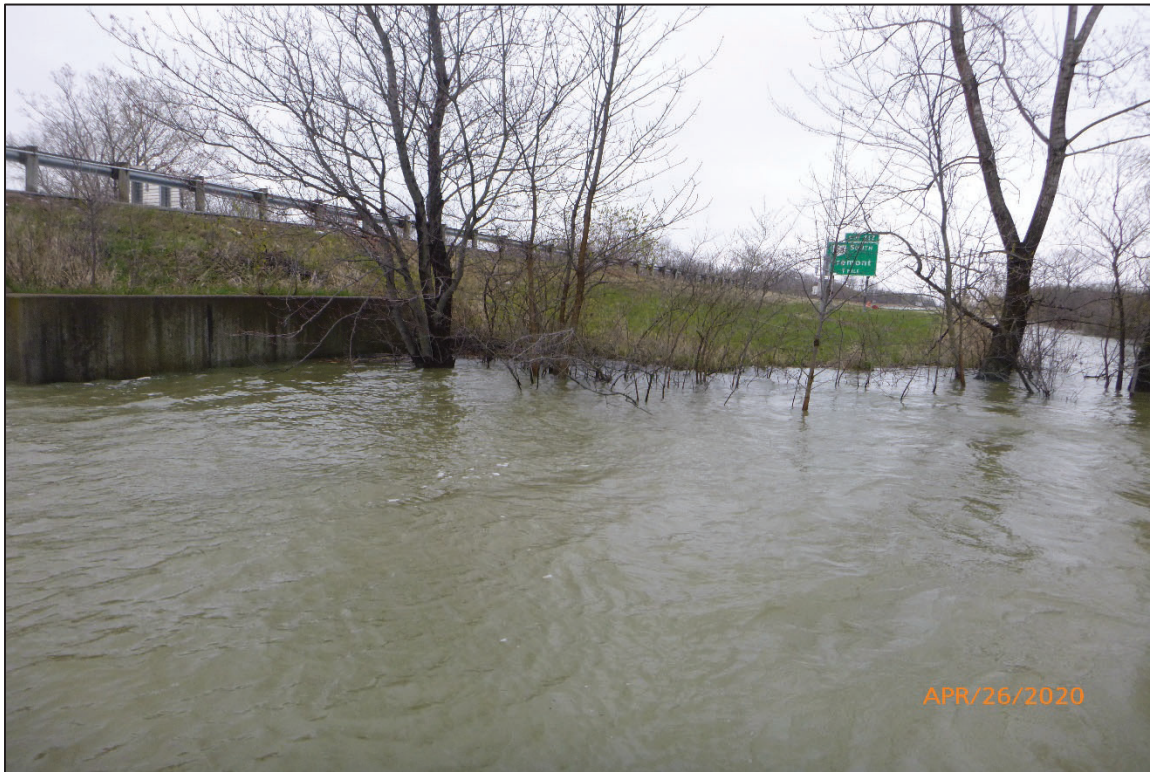
Photograph No. 5: View of the East Embankment Upstream of the Structure, Looking Northeast.
