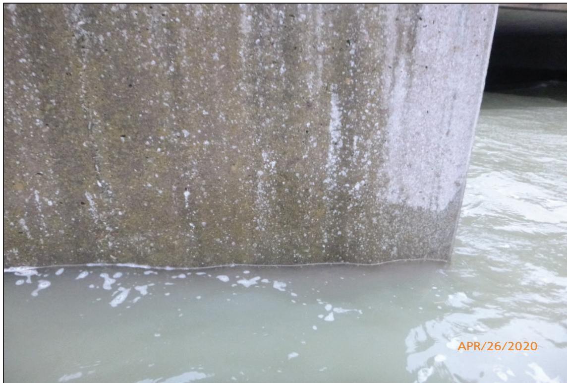
Photograph No. 11: View of the Typical Concrete Condition at the Waterline on the South Corner of Abutment 1, Looking North.
