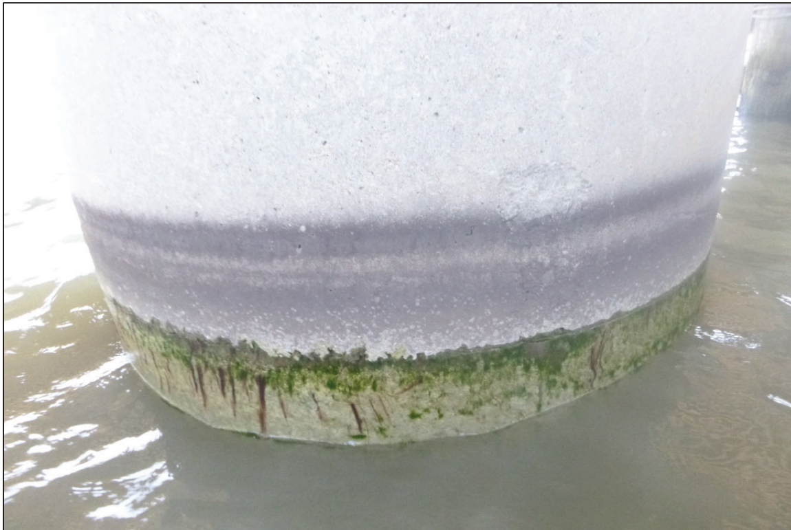
Photograph No. 54: View of the Typical Concrete Condition at the Waterline of an Original Column design on the North Face of Bent 1, Looking South.
