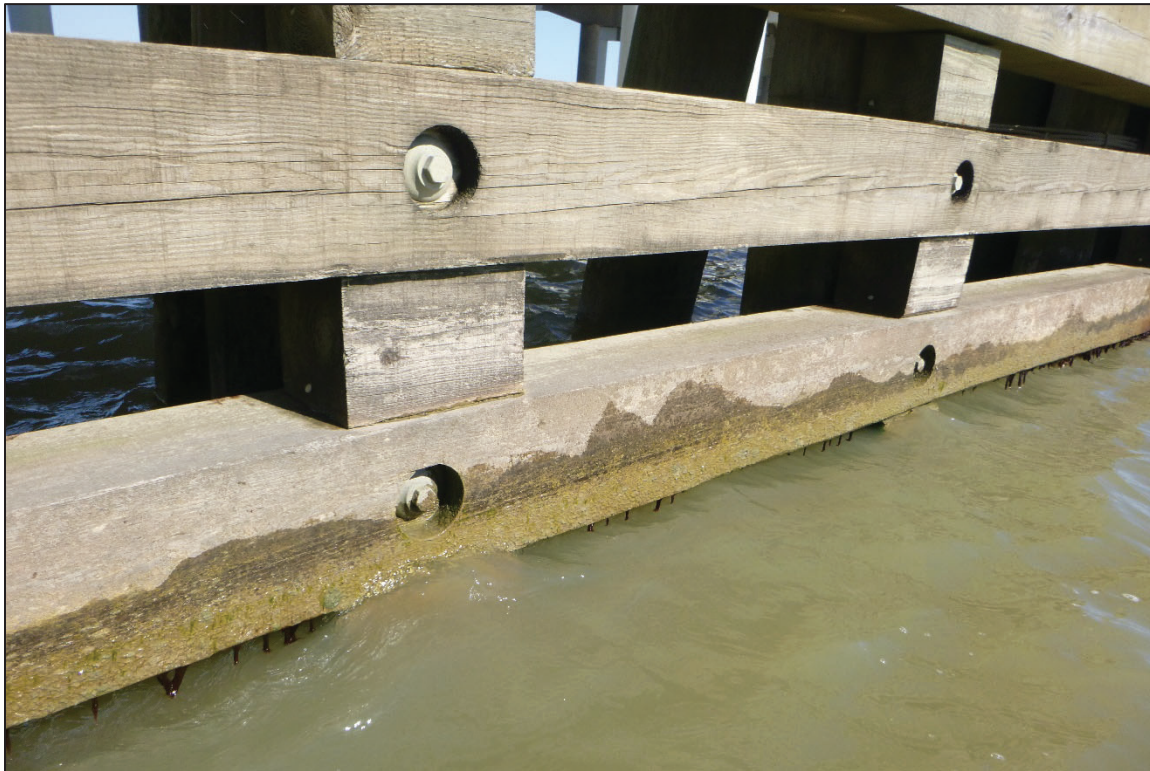
Photograph No. 58: View of the Typical Fender of the Fender System, Looking Northeast.
