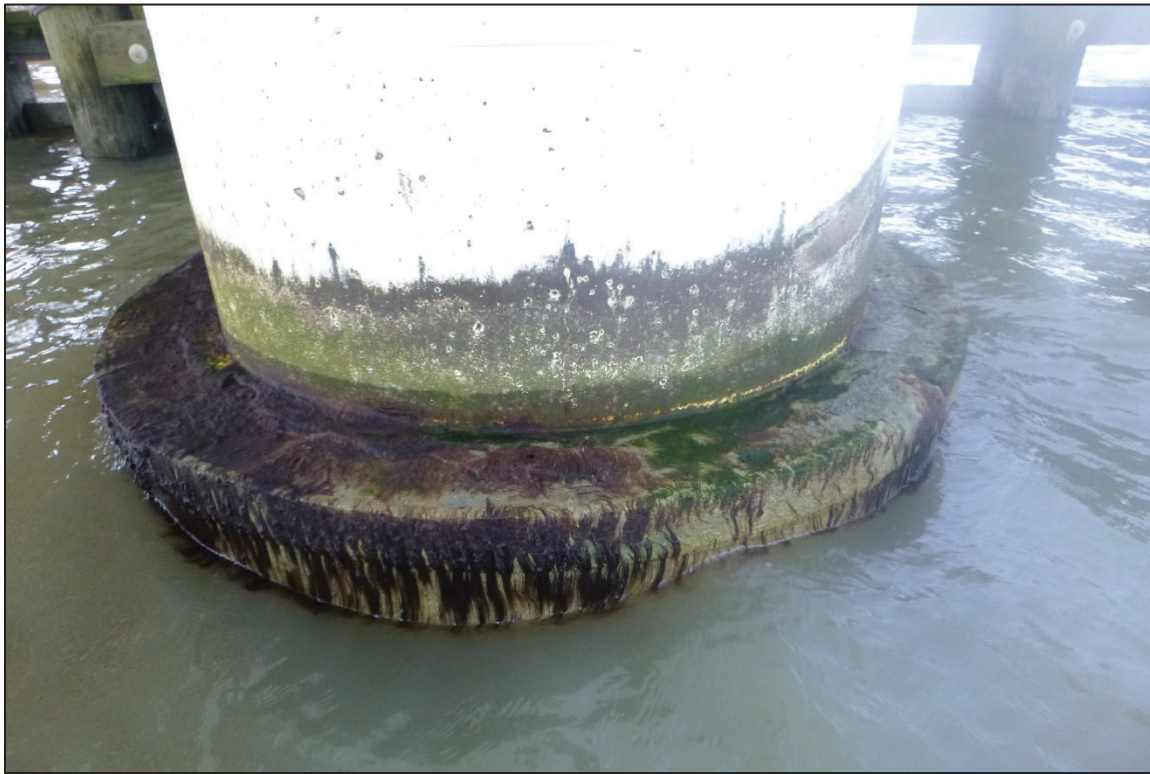
Photograph No. 53: View of the Typical Concrete and Steel Condition at the Waterline of a New Column design on the North Face of Bent 1, Looking South.
