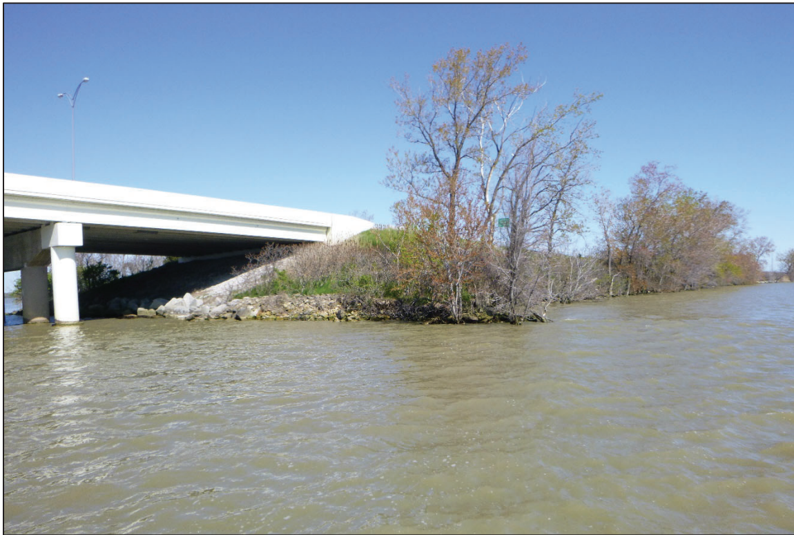
Photograph No. 5: View of the North Embankment Downstream of the Structure, Looking Northwest.
