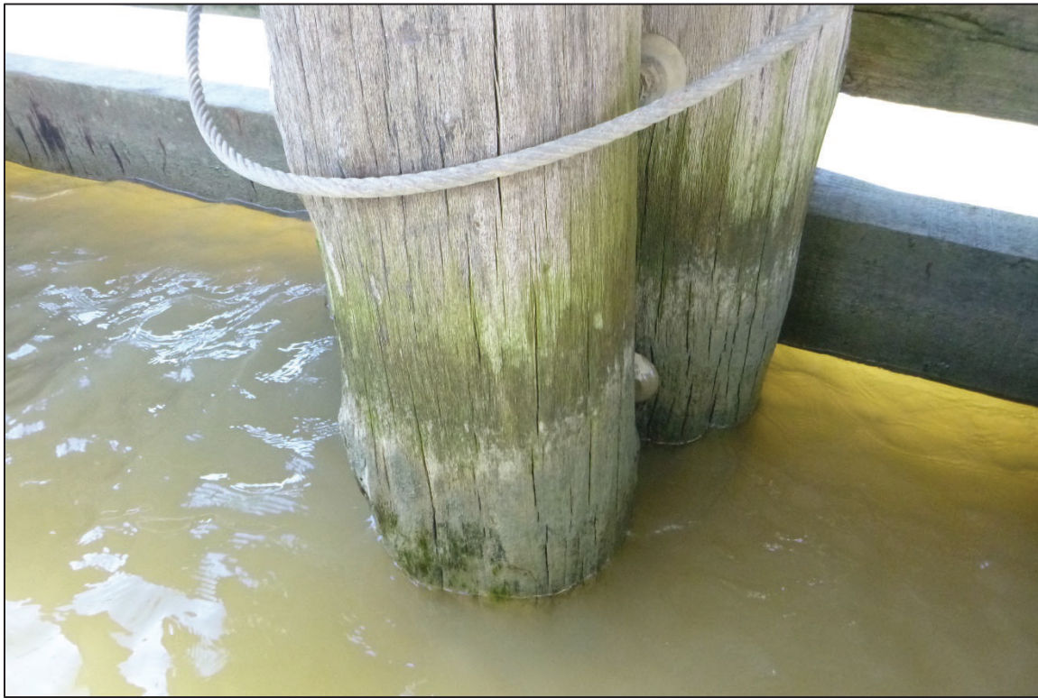
Photograph No. 57: View of the Typical Timber Pile of the Fender System, Looking Southeast.
