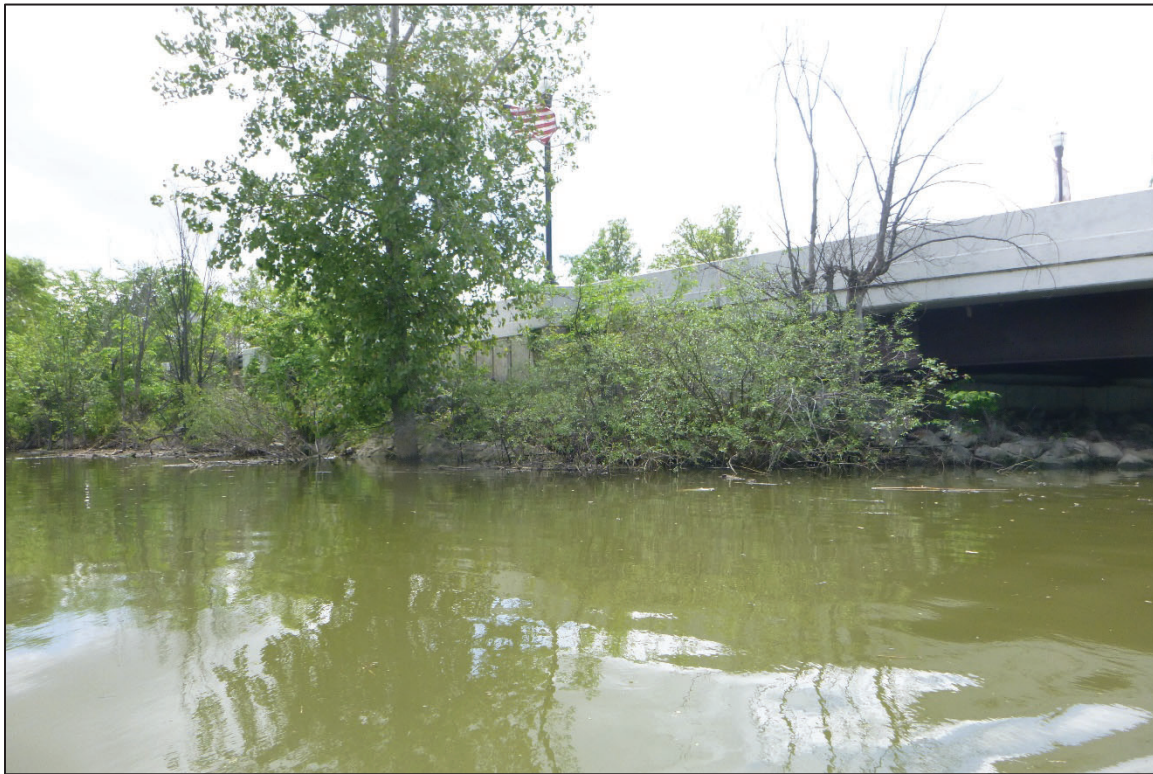
Photograph No. 5: View of the North Embankment Downstream of the Structure, Looking Southwest.
