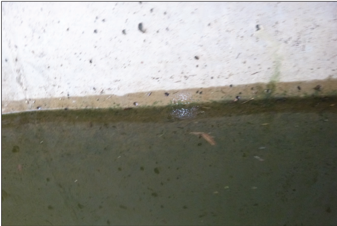
Photograph No. 17: View of the Typical Concrete Condition at the Waterline on the South Face of Pier 4.
