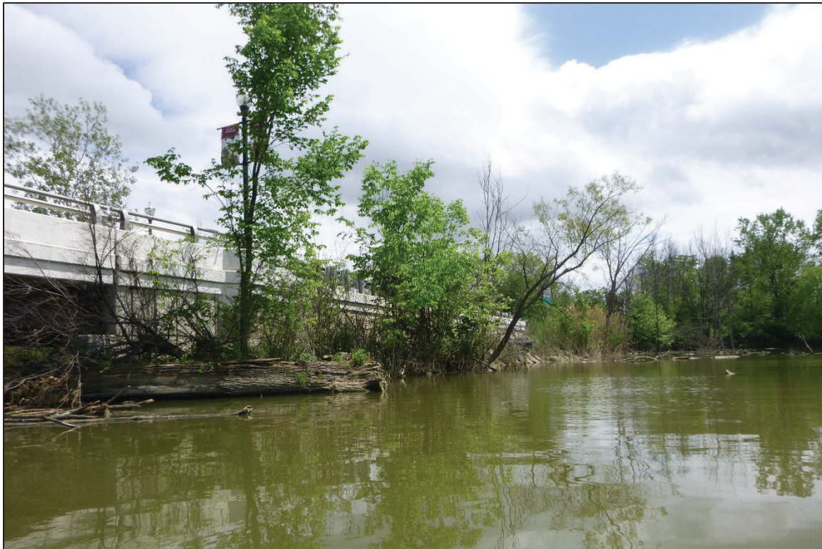
Photograph No. 6: View of the South Embankment Upstream of the Structure, Looking Southeast.
