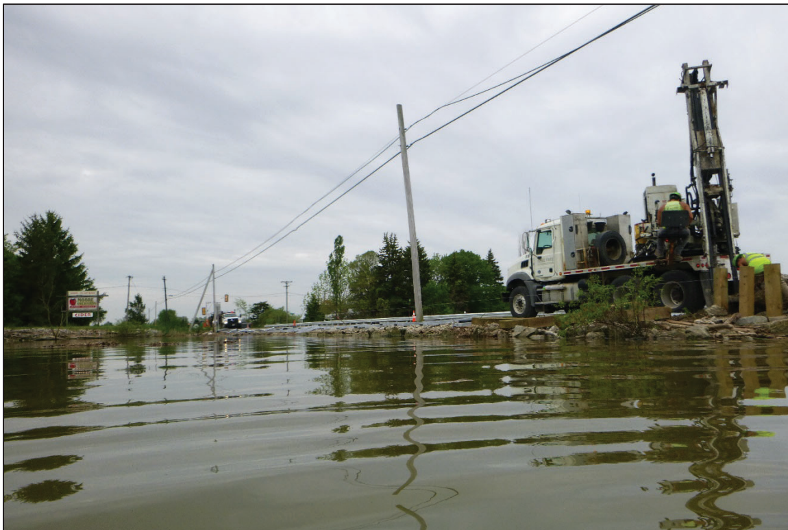
Photograph No. 6: View of the South Embankment Downstream of the Structure, Looking Southwest.
