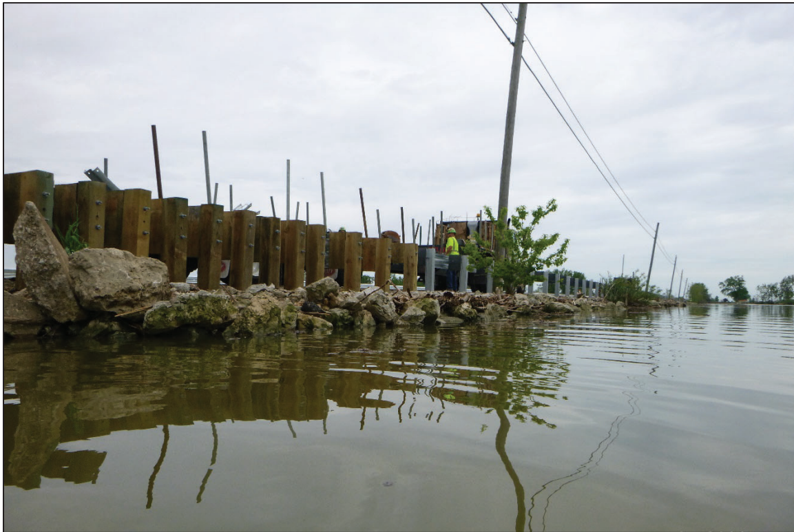
Photograph No. 4: View of the North Embankment Downstream of the Structure, Looking Northwest.
