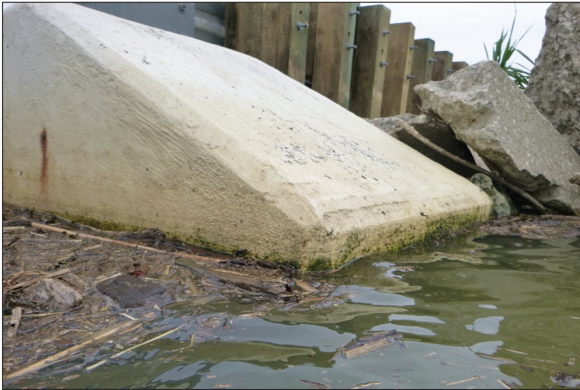
Photograph No. 7: View of the Typical Concrete Condition at the Waterline, Looking Northwest.
