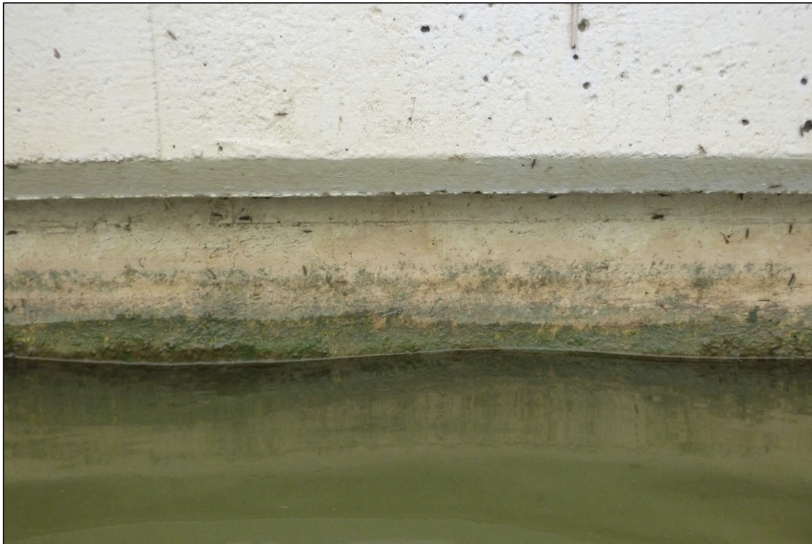
Photograph No. 8: View of the Typical Concrete Condition at the Upstream Nose of Pier 1 at the Waterline, Looking East.
