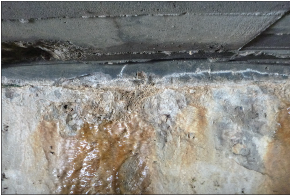
Photograph No. 7: View of the Typical Concrete Condition of the Abutments at the Waterline, Looking North.
