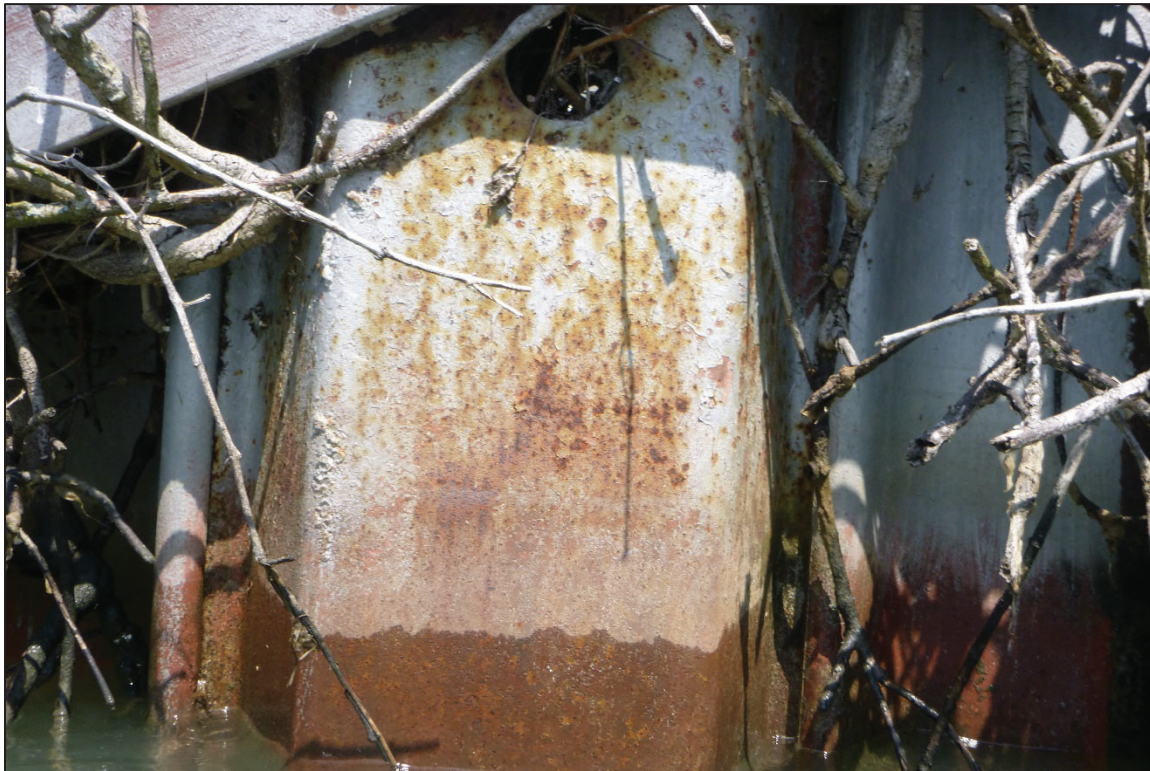
Photograph No. 12: View of the Typical Steel Condition at the Waterline on the Abutment 2, Looking North.
