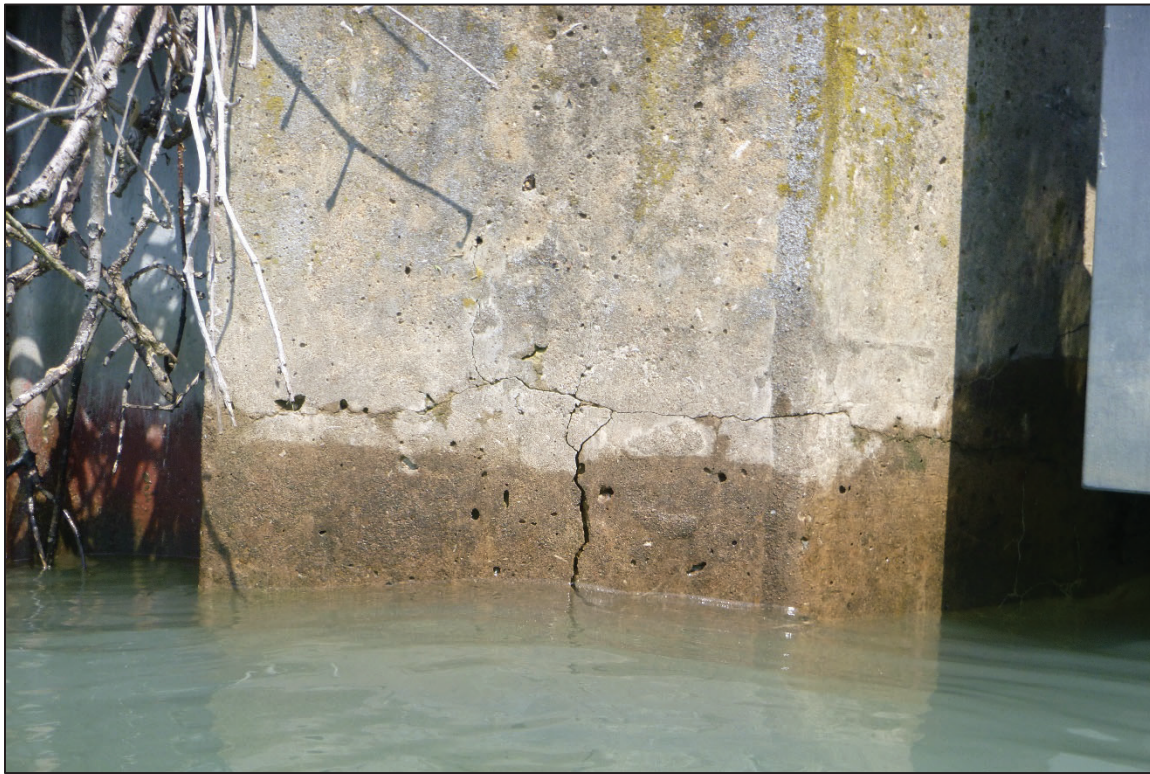
Photograph No. 11: View of the Typical Concrete Condition and Crack at the Waterline on the Abutment 2, Looking North.
