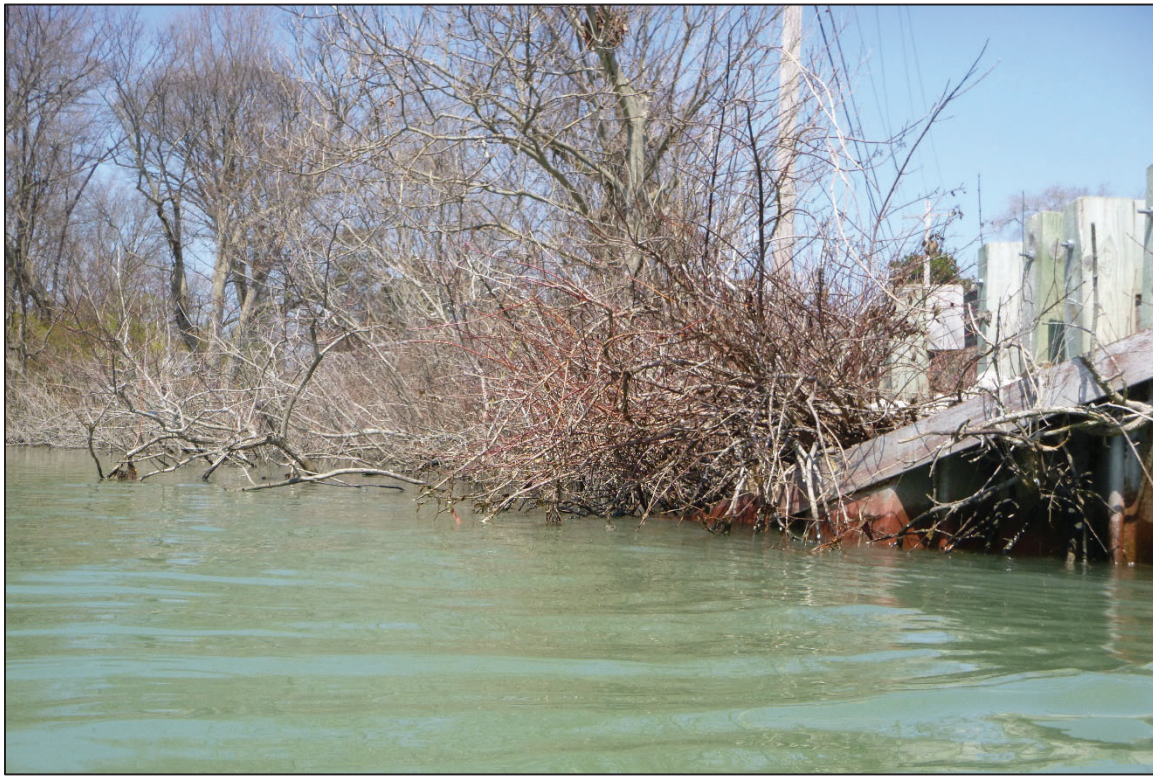
Photograph No. 3: View of the North Embankment Upstream of the Structure, Looking North.
