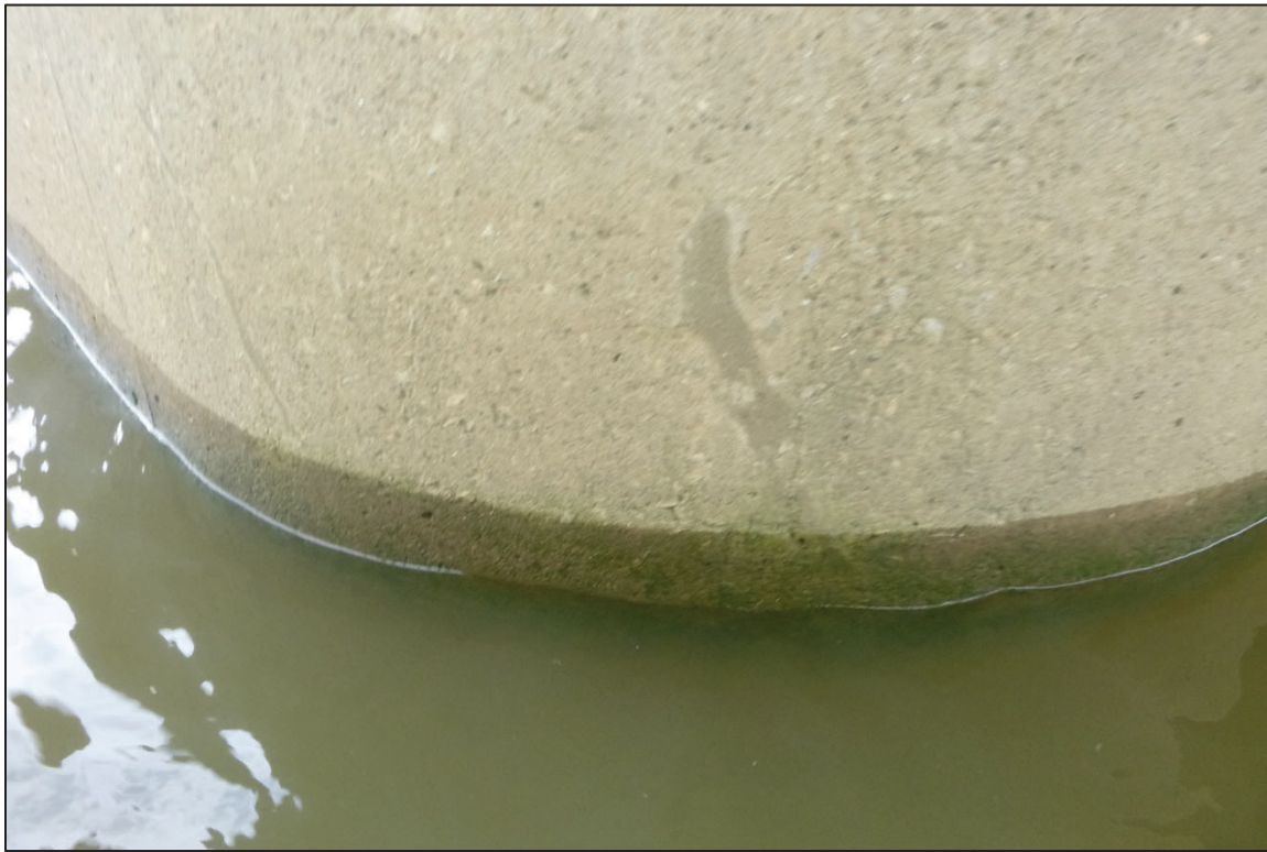
Photograph No. 11: View of the Typical Concrete Condition at the Waterline on the Upstream Nose of Pier 4, Looking West.
