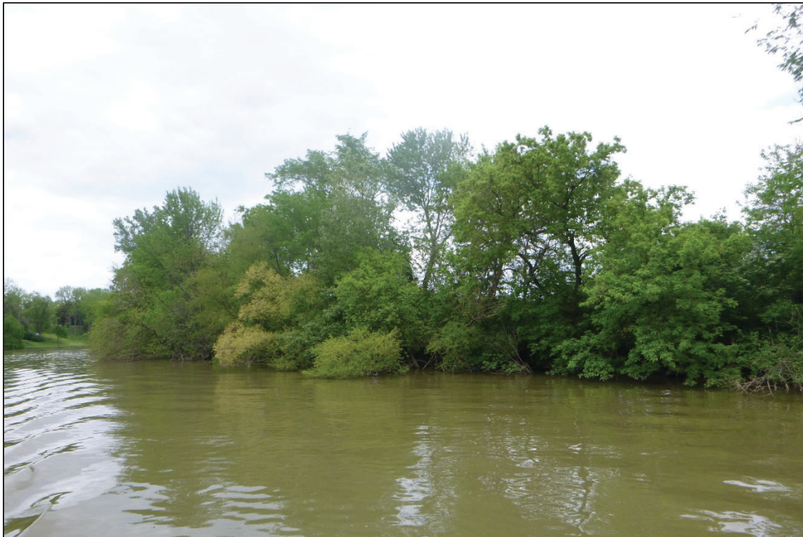
Photograph No. 8: View of the East Embankment Downstream of the Structure, Looking Northeast.
