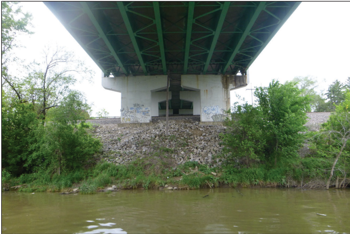
Photograph No. 4: View of the West Embankment at the Structure, Looking West.
