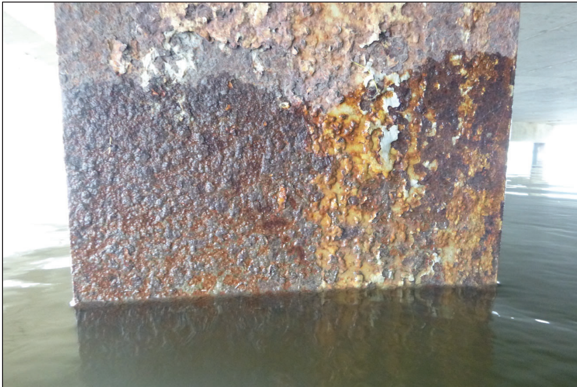
Photograph No. 18: View of the Typical Steel Condition at the Waterline on the Upstream Nose of Bent 1, Looking South.
