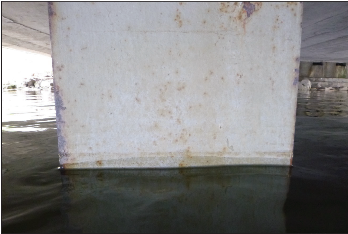
Photograph No. 17: View of the Typical Steel Condition at the Waterline on the Bent 4, Looking North.
