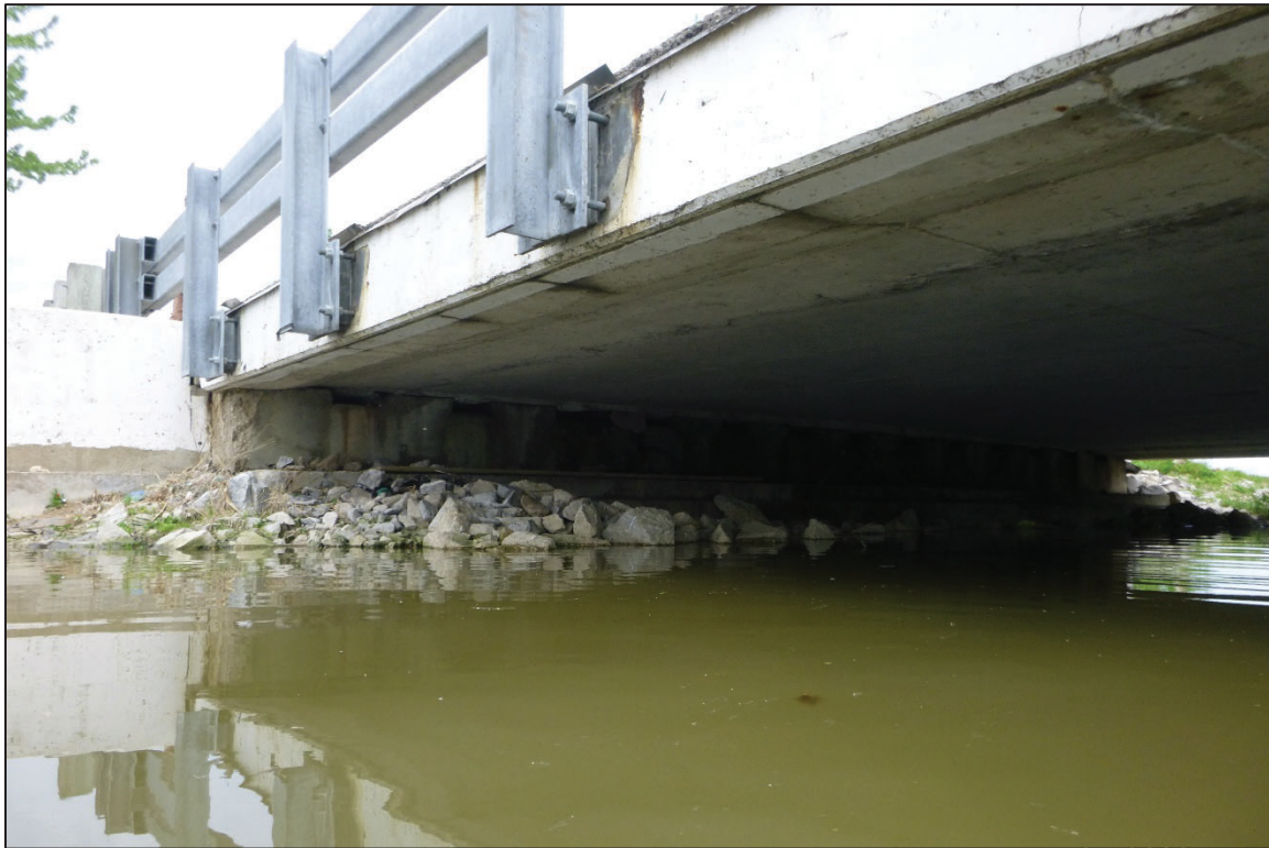
Photograph No. 4: View of the North Embankment at the Structure, Looking Northeast.
