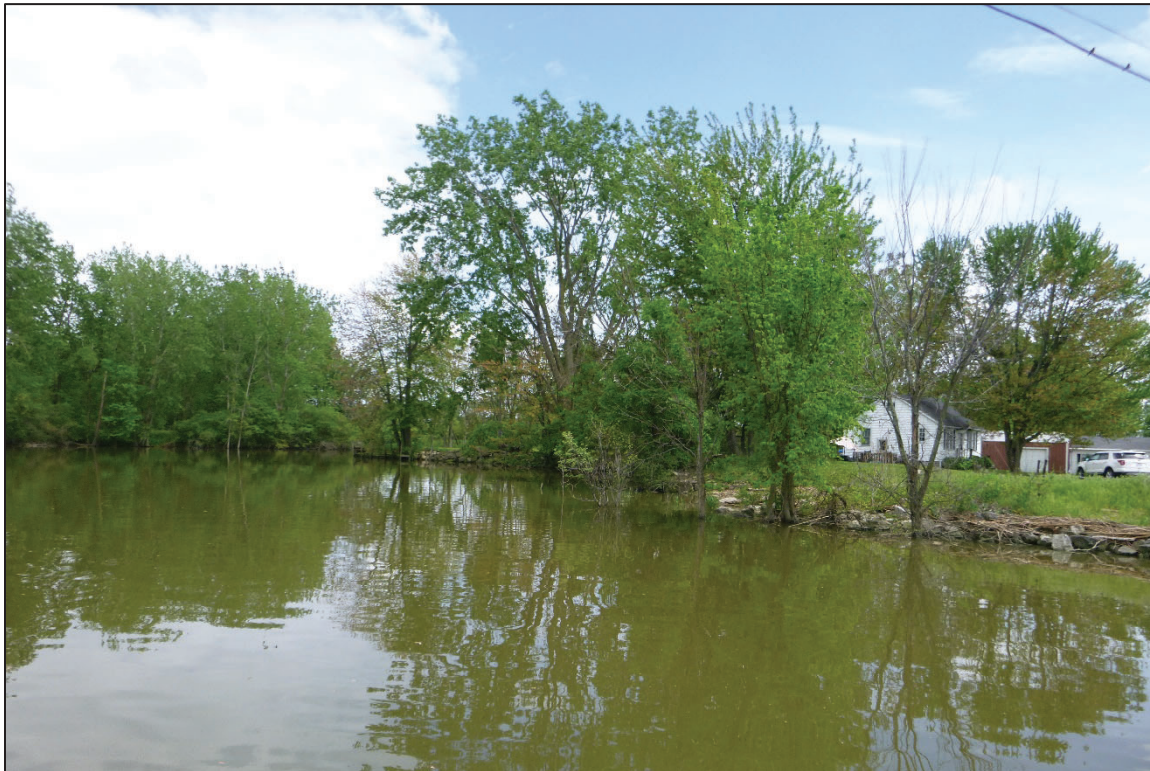
Photograph No. 8: View of the South Embankment Downstream of the Structure, Looking Southeast.
