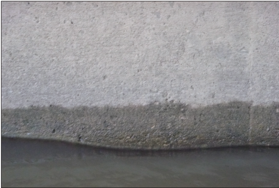
Photograph No. 17: View of the Typical Concrete Condition at the Waterline, Looking West.
