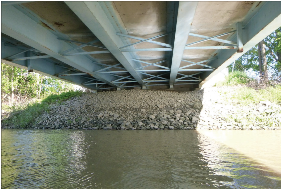
Photograph No. 7: View of the East Embankment at the Structure, Looking East.
