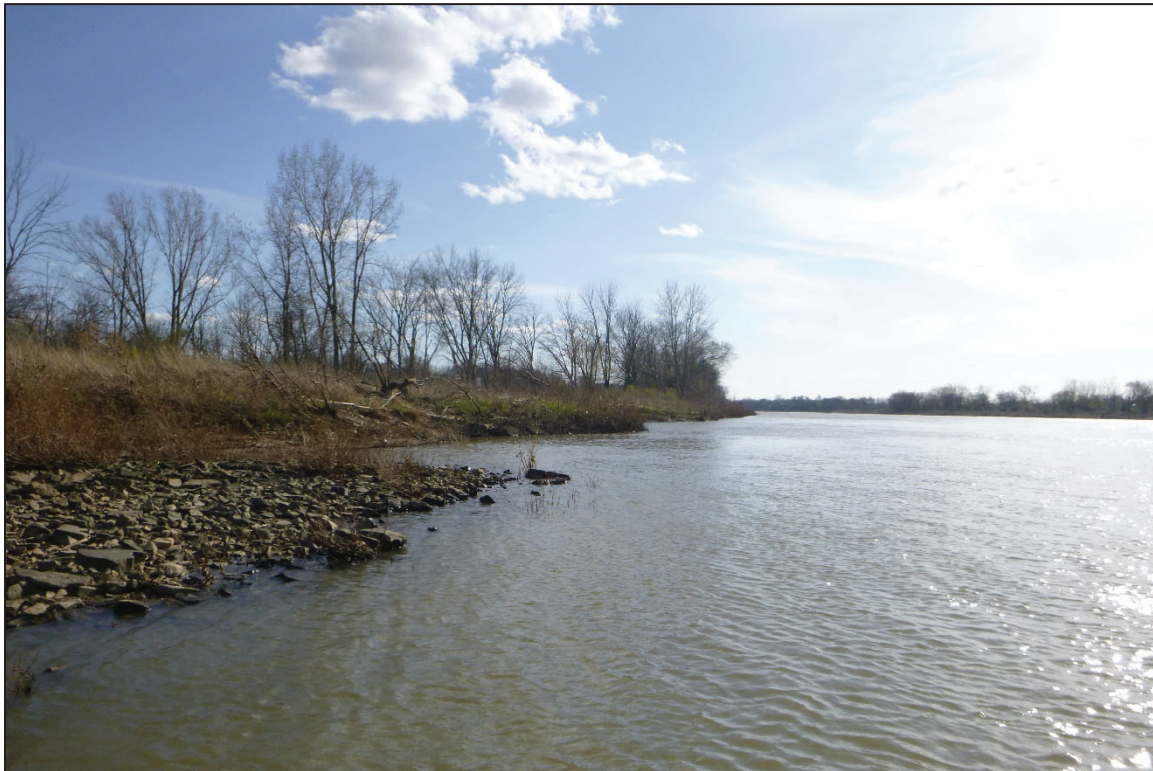
Photograph No. 6: View of the South Embankment Upstream of the Structure, Looking West.
