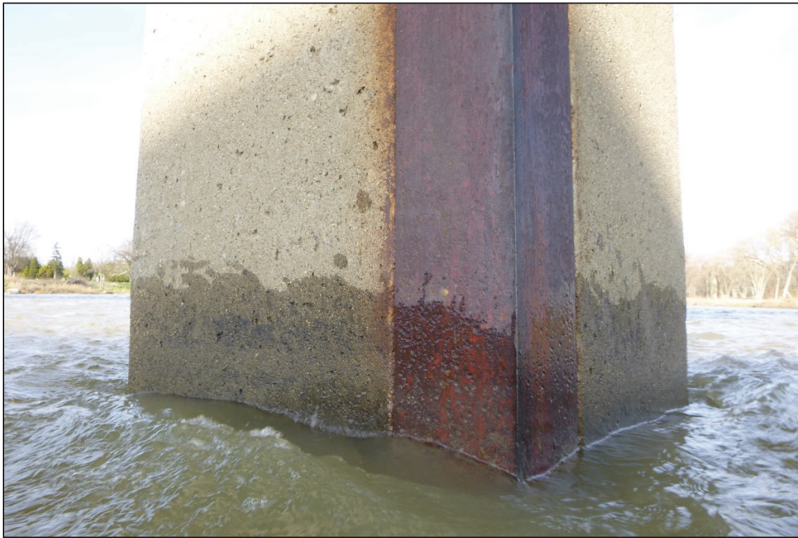
Photograph No. 17: View of the Typical Concrete and Steel Icebreaker Condition at the Waterline, Looking East.
