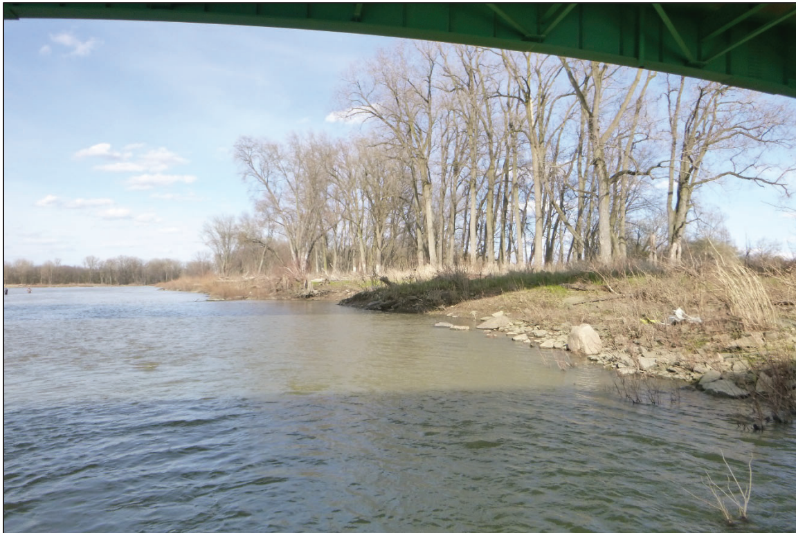
Photograph No. 8: View of the South Embankment Downstream of the Structure, Looking East.
