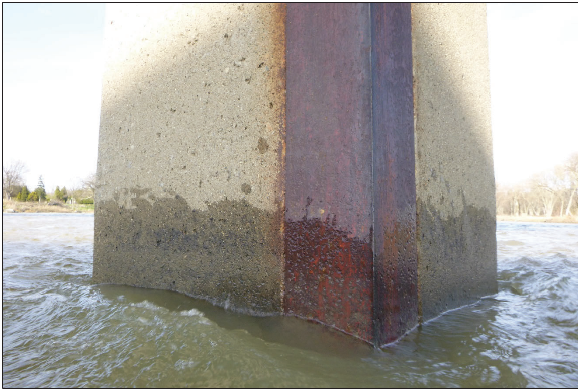
Photograph No. 17: View of the Typical Concrete and Steel Condition at the Waterline, Looking East.
