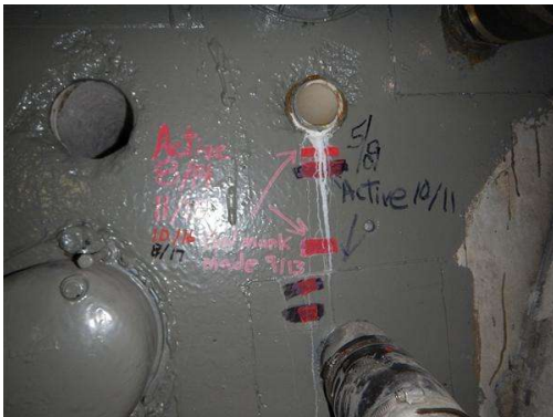
Photo 15 Active efflorescence in the diaphragm at Pier 2Z.
