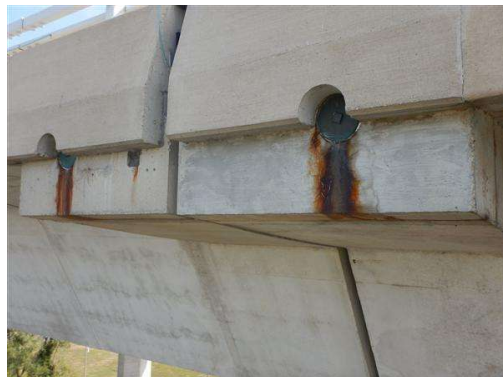
Photo 12 Heavy rust staining and efflorescence on the edge face of the end segments.
