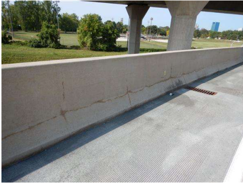
Photo 7 Moderate vertical and horizontal cracking and efflorescent leaching along the west parapet.
