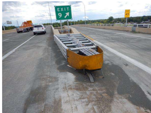
Photo 10 Damaged attenuator at the Ramp Z exit.
