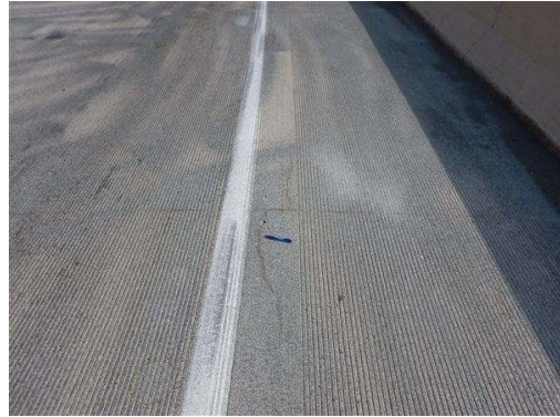
Photo 2 Typical longitudinal crack in the shoulder of the deck in Span 20Z.
