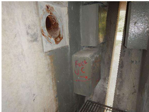
Photo 3 Delaminated concrete at the PT end blockout at Pier 15Z.
