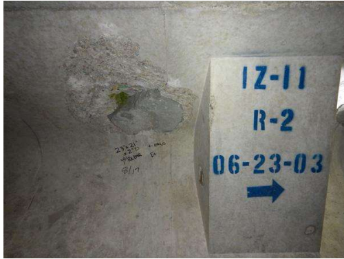
Photo 1 Lift hole with spalled concrete and exposed reinforcement and efflorescence in Span 1Z.
