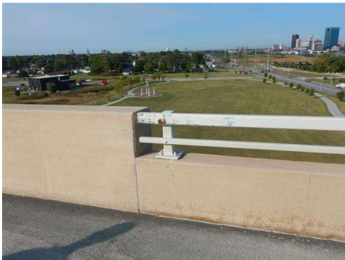
Photo 9 Collision damage to the concrete and steel railings in Span 6Z.
