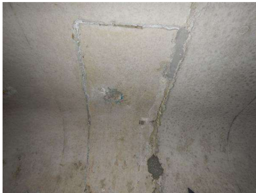
Photo 3 Typical lift hole condition and construction joint with efflorescence.
