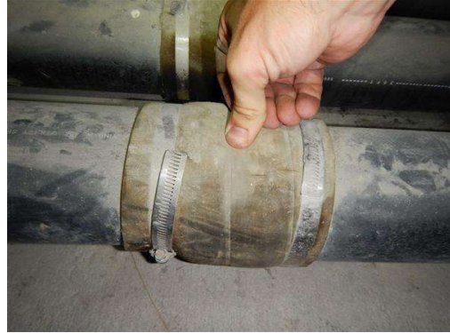
Photo 8 Weakened grout within the coupler between tendon ducts in Span 1Z.
