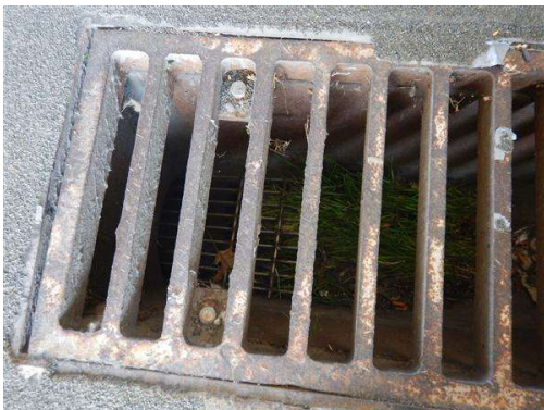
Photo 11 Partially filled scupper with displaced grate within the element.
