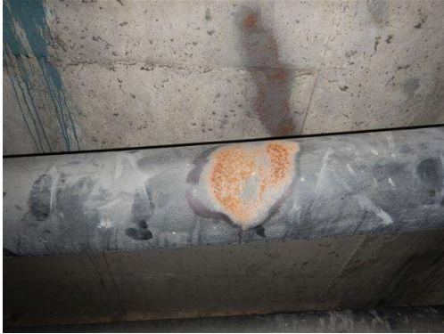
Photo 7 Typical rust deposit on the PTFE tendon sheathing.
