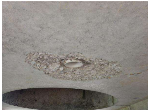
Photo 4 Spalled concrete on the exterior bottom flange of the box segment in Span 16Z.
