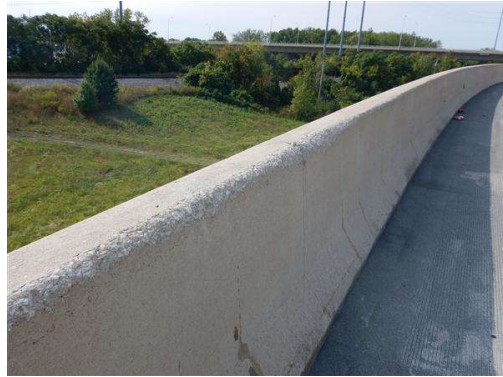
Photo 8 Scaling along the top edge of the west parapet in Span 24Z.
