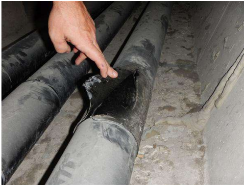
Photo 9 Splice material not properly adhered to the PTFE tendon sections in Span 23Z.
