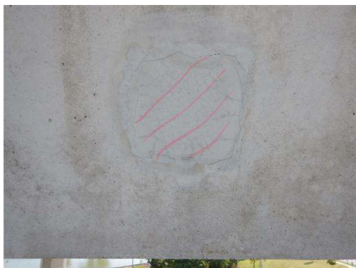
Photo 5 Delaminated patch on the exterior web of the box segment in Span 2Z.
