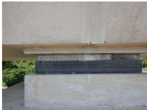
Photo 18 Spalled concrete in the plinth of the east bearing at Pier 5Z.
