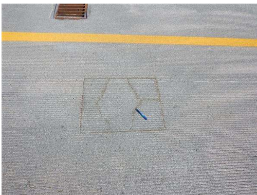
Photo 5 Delaminated and unsound patch with map cracking located in Span 17Z.
