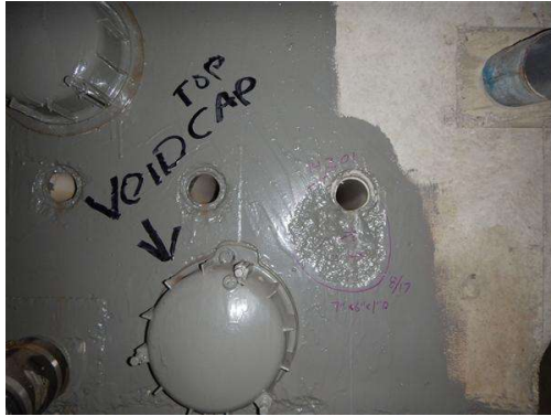
Photo 1 Small void noted in the T2 tendon end cap at Pier 14Z.
