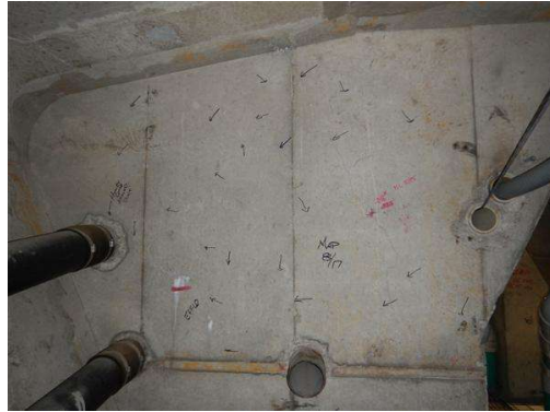
Photo 14 Area of map cracking ranging in width from hairline to 0.016 in. with efflorescence in diaphragm at Pier 21Z.
