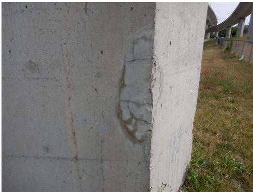
Photo 3 Delaminated area and cracking in the pier column concrete at Pier 9Z.
