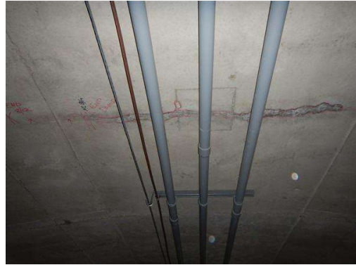
Photo 8 Transverse hairline crack in the top slab of the interior box segment with inactive efflorescence and discoloration.
