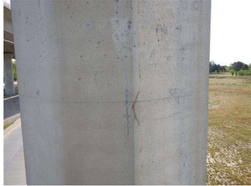
Photo 2 Typical narrow vertical cracks in the pier columns.
