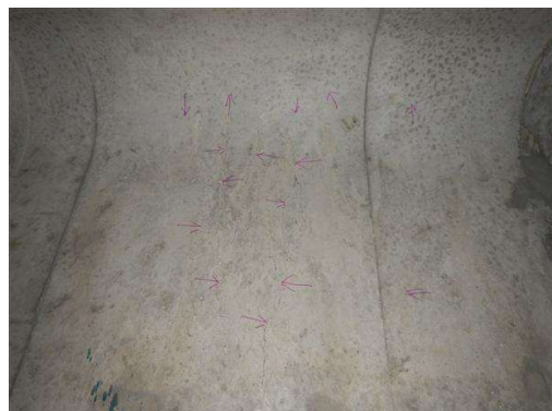
Photo 6 Area of hairline map cracking in the interior web of the box segment in Span 12Z.
