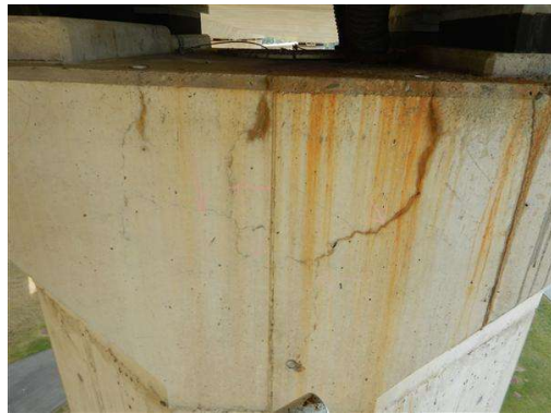
Photo 4 Typical cracking and efflorescence/staining in the pier caps.
