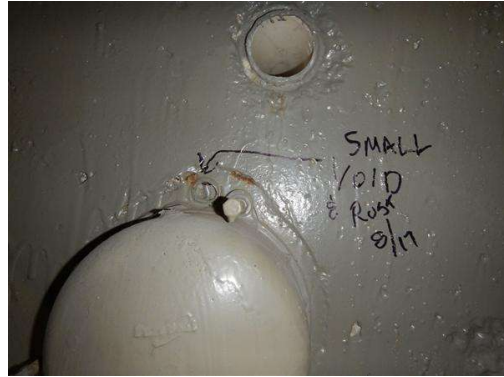
Photo 2 Small void in the grout tube and rust present on the T2 tendon duct located at Pier 20Z.
