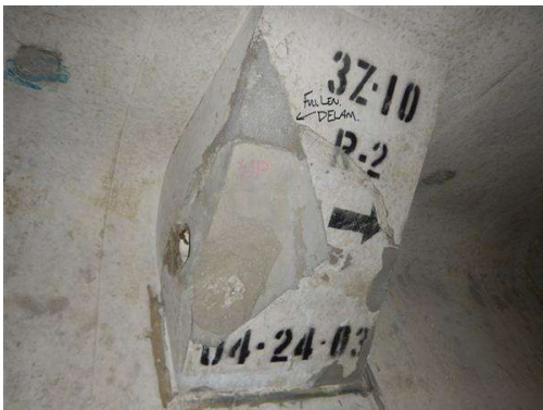
Photo 11 Delaminated area on exterior stressing block in Span 3Z.
