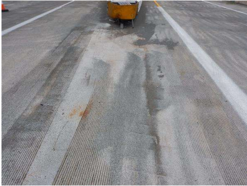
Photo 1 Longitudinal joint with map cracking and efflorescent leaching over the length.
