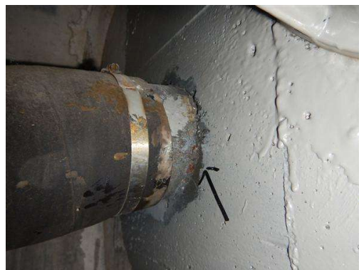
Photo 6 Rust present on the PT duct and clamps at the diaphragm connection at Pier 7Z.
