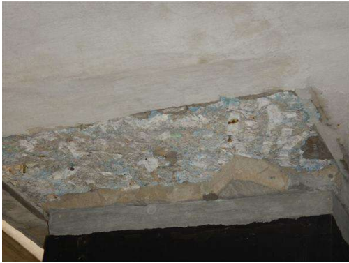
Photo 19 Spalled concrete in the plinth with exposed reinforcement at the western bearing at Pier 12Z.
