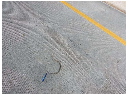
Photo 4 Typical top of deck lift hole patches with cracking and spalling.
