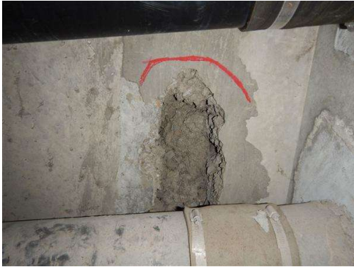
Photo 13 Area of poorly consolidated concrete in the closure pour joint at Pier 15Z.
