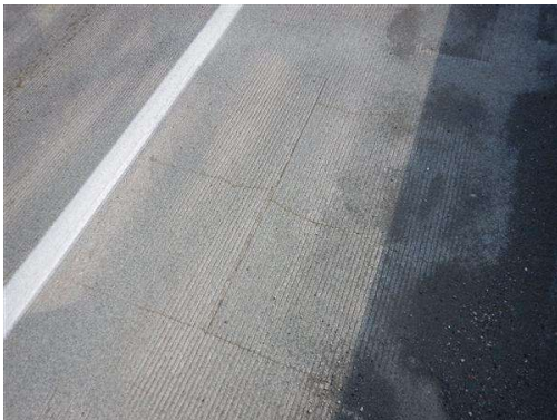
Photo 3 Map cracking in the shoulder of the deck in Span 19Z.
