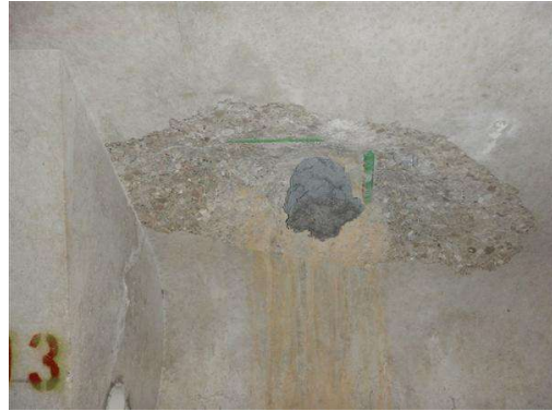
Photo 2 Severe spall at lift hole location with exposed reinforcement in Span 1Z.
