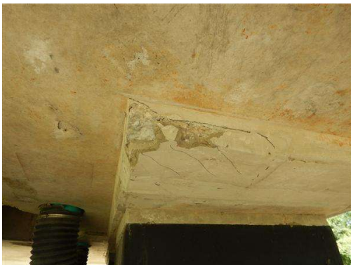
Photo 17 Spall and delaminated concrete in the southeast plinth at Pier 4Z.
