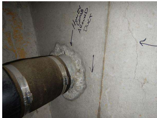
Photo 16 Honeycombed concrete around the PT duct in the diaphragm at Pier 21Z.
