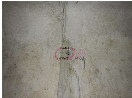
Photo 10 Typical void at the interior construction joint of the box segment.
