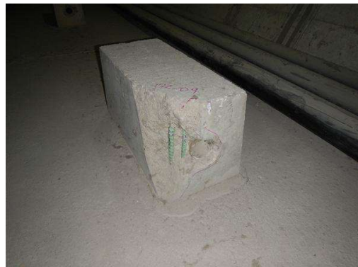
Photo 12 Bottom exterior stressing block with spalled concrete and exposed reinforcement.
