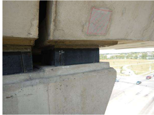
Photo 20 Missing patch pin groove strips on both Pier 21Z elastomeric bearings.
