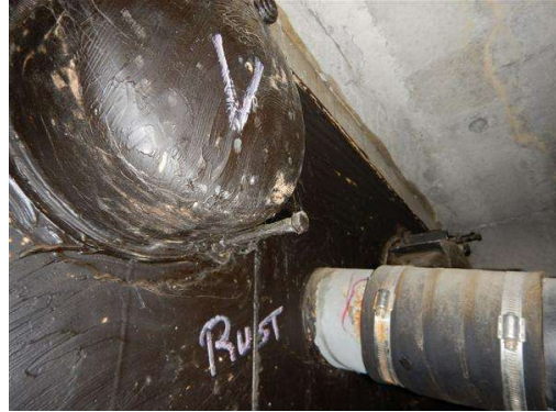
Photo 2 Small voids in PT caps and PT clamp and duct rusting at Pier 1A looking Southwest
