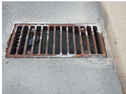
Photo 12 Scuppers clogged with debris on the west side of the bridge between Spans 4A & 5A
