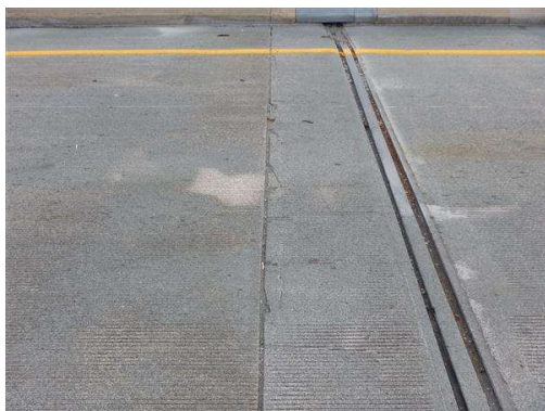
Photo 17 Concrete spalls in the header at the expansion joint at Abutment 1A looking West
