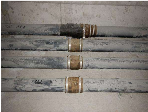
Photo 3 Bulging PT ducts
