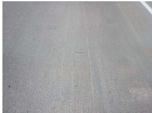
Photo 4 Longitudinal cracks in the wearing surface
