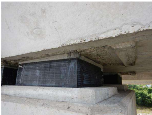
Photo 17 Concrete spall on the West bearing, SW Corner at Pier 7A
