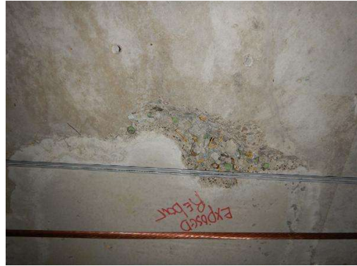
Photo 2 Concrete spall in the top flange slab with rebar exposed in Span 10A, Segment 04
