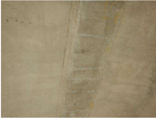
Photo 1 Bottom of the deck slab closure pour transverse cracks exhibiting efflorescence between Spans 15A & 16A looking South
