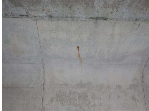
Photo 2 Rust stains on the deck slab looking West
