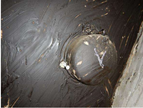
Photo 1 Bolt missing and noted void in PT anchor cap at Pier 1A.
