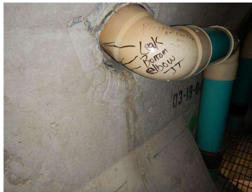
Photo 14 Interior drainage pipe at Pier 4A, rust staining
