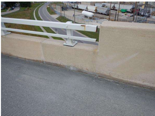
Photo 11 At the barrier transition, minor rust on steel railing and map cracks in barrier in Spans 7A & 8A looking West
