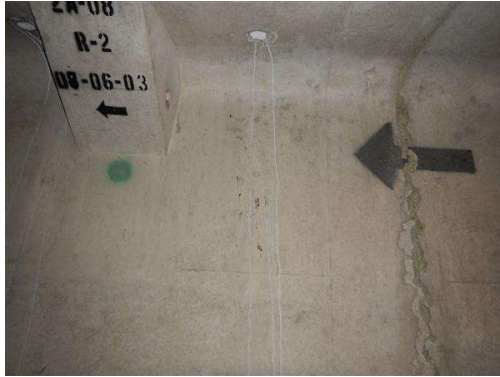
Photo 1 Leaching efflorescence from lift holes in Span 2A looking West
