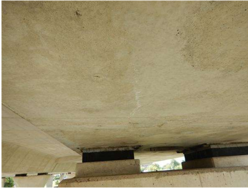
Photo 7 Longitudinal cracks with efflorescence in the bottom flange near Pier 8A
