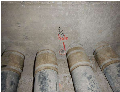
Photo 15 Form-tie hole at Pier 15A not fully grouted
