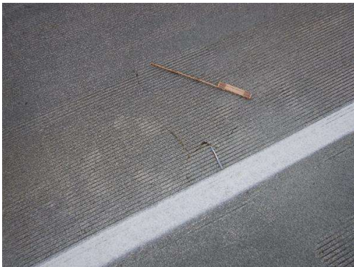
Photo 3 Transverse and map cracks in the wearing surface between Spans 4A & 5A
