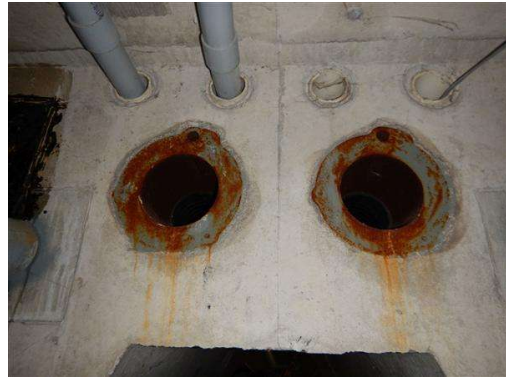
Photo 4 Typical moderate rust on the future PT ducts located in the diaphragms at Pier 1A
