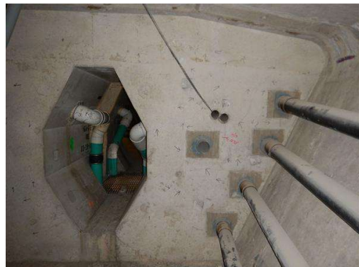
Photo 12 Map cracks ranging from 0.016" to 0.030" with efflorescence on the Pier 17A Diaphragm
