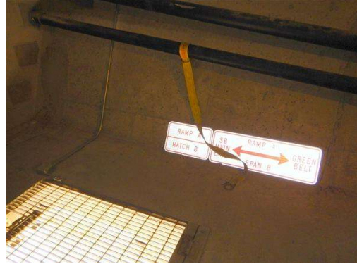
Photo 2 Safety lanyard attached to the PT duct at Pier 8A
