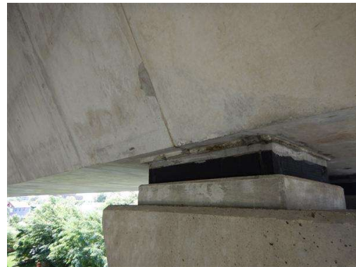
Photo 16 Cracks and delaminated concrete in the plinth of Pier 12A East bearing
