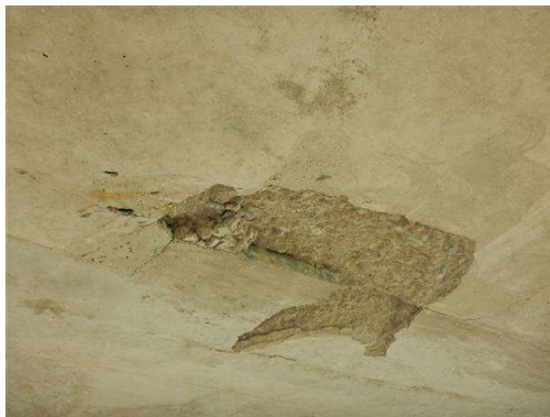
Photo 5 Concrete spall with rebar exposed in the bottom flange of Span 15A, Segment 12
