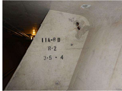
Photo 14 Concrete spall in diaphragm at Segment 8D in Span 11A, measuring 16"x12"x3/4",
