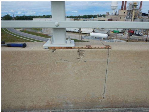
Photo 9 Delaminated concrete under the steel railing in Spans 8A & 9A looking West
