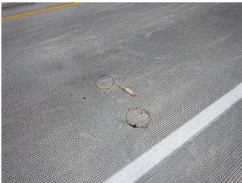
Photo 5 Concrete patches with spalls and discoloration between Spans 4A & 5A
