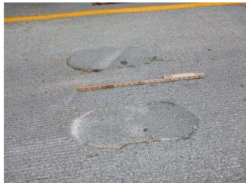
Photo 6 Depressed concrete patches at Spans 3A & 4A
