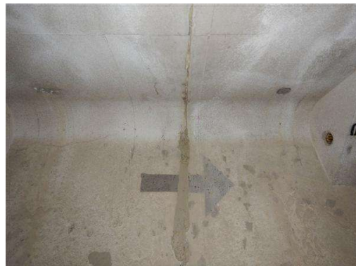
Photo 6 Typical hairline horizontal cracks with efflorescence in the interior segment at Pier 4A
