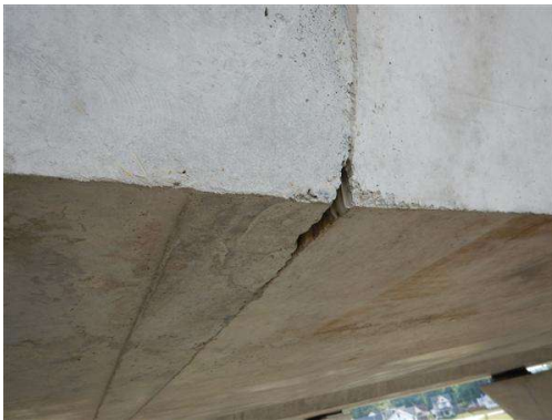
Photo 9 Void in the bottom flange between Segments 10A & 11A in Span 14A
