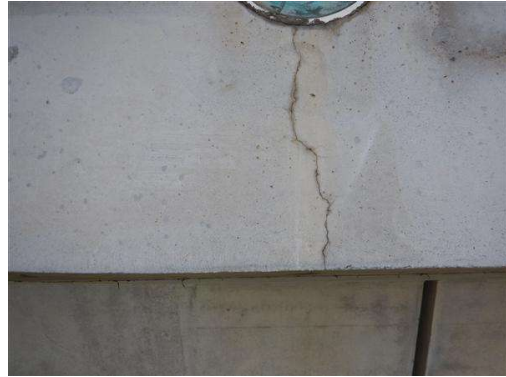
Photo 8 Cracks in exterior pier segment at Pier 17A on the West side looking East
