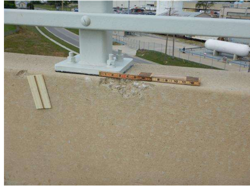
Photo 8 Concrete spall under steel railing in Spans 8A & 9A looking West
