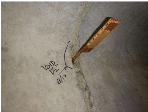
Photo 11 Void in web segment joint at Segment 5A in Span 1A.
