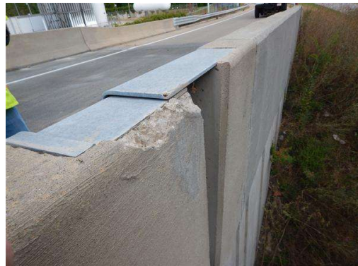
Photo 10 Concrete spall on the East parapet at Abutment 1
