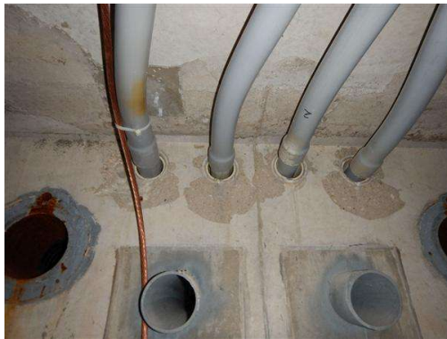
Photo 3 Concrete spalls around the ducts at the Pier 13A
