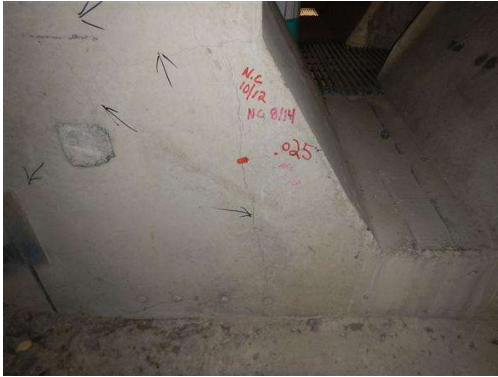
Photo 13 Typical cracks in the vertical face of the interior diaphragm at Pier 9A
