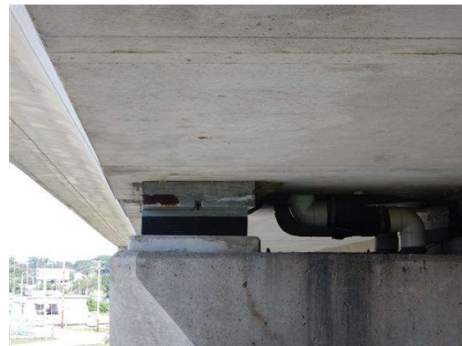
Photo 18 Steel sliding plate with rust at the Pier 11A west bearing
