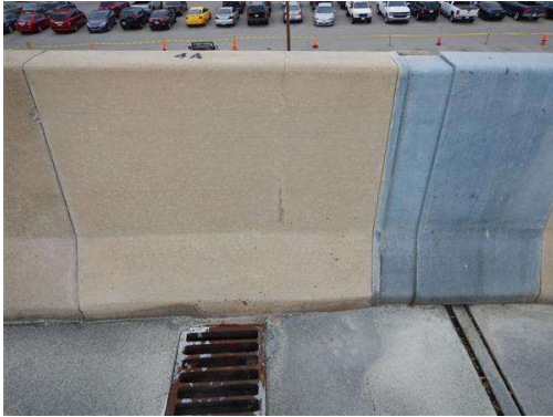
Photo 7 Horizontal and vertical cracks in the concrete parapet in the Spans 4A & 5A looking West
