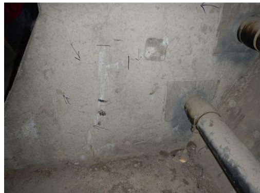
Photo 12 Typical cracking on the vertical face of the interior diaphragm.
