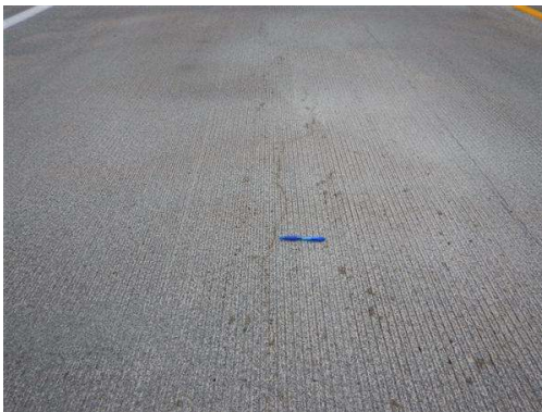
Photo 5 Typical longitudinal and map cracks located in the middle of the travel lane in Span 10D.
