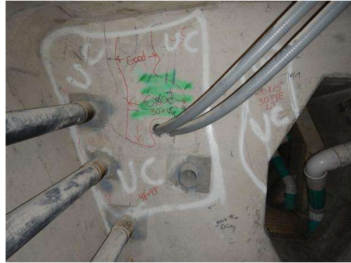
Photo 14 Area of delaminated concrete and cracking on the diaphragm at Pier 3D.
