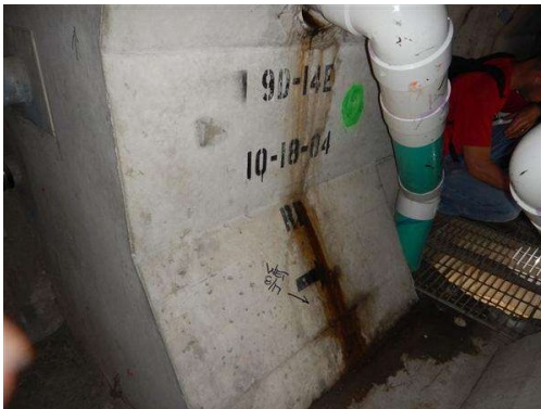
Photo 15 Interior drainage pipe at Pier 1D with wet concrete, rust staining and efflorescence.
