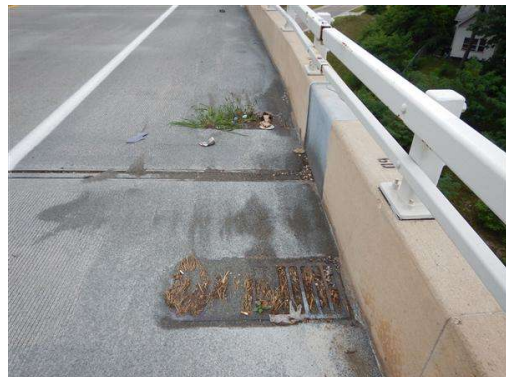
Photo 12 Heavy debris and vegetation present in the deck scuppers at Pier 7D.
