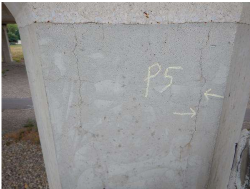
Photo 3 Typical hairline to medium width vertical and map cracks on the pier columns.
