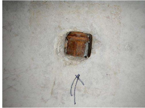
Photo 2 Large bolt encased in the lift hole concrete with the hole not patched.
