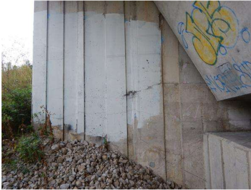
Photo 1 Typical horizontal and map cracking along the full height of the Abutment 13D backwall.
