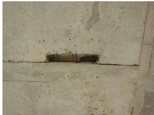
Photo 10 Typical exterior void between segment joints.
