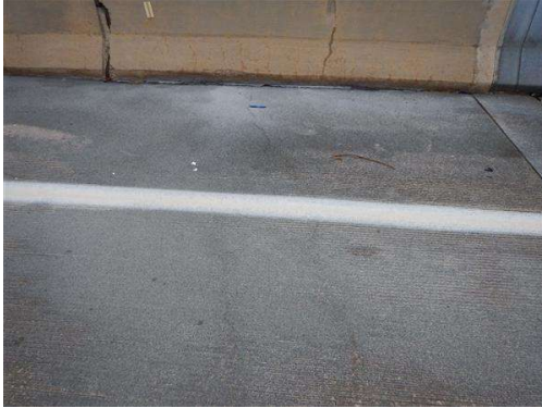
Photo 1 Moderate transverse cracking in the approach slab running full width.
