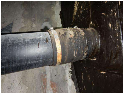
Photo 3 Typical rust on clamps connecting PT ducts with sheathing.
