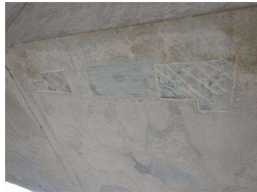
Photo 4 Delaminated concrete at exterior hold down patch in the bottom flange of Span 6D.
