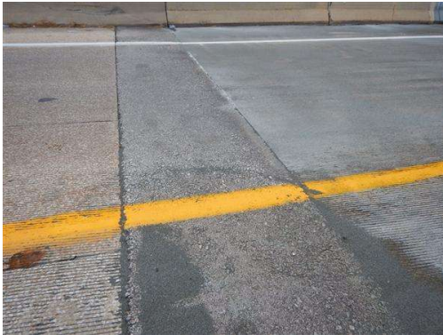
Photo 3 Typical condition of the relief joint at the end of the approach slab.
