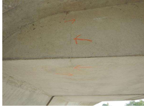
Photo 8 Typical cracking along the width of the end pier segment flanges.
