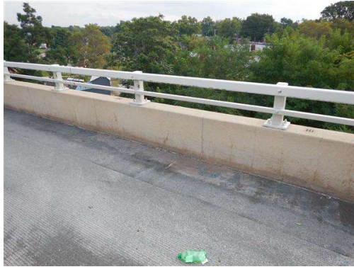
Photo 7 Typical vertical cracking and discoloration in the concrete parapet along the length of the bridge.
