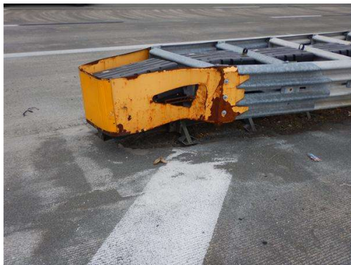
Photo 11 Collision damage to the attenuator at the Ramp D exit.
