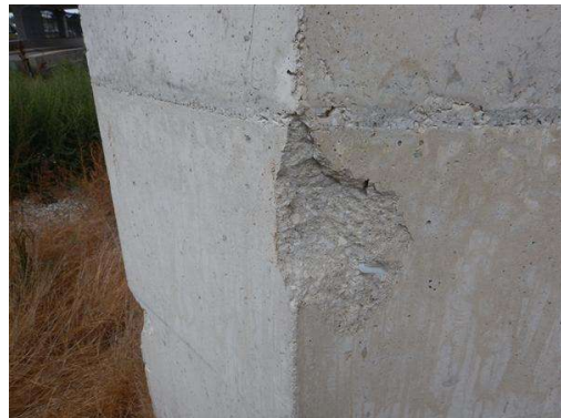
Photo 4 1 ft. x 1 ft. x 2.5 in. deep spall near ground level on the Pier 9D column.
