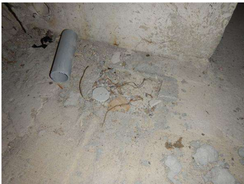
Photo 11 Hold down hole in the bottom flange of the Span 2D segment partially filled with grout.
