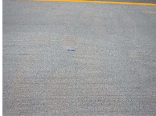
Photo 2 Typical transverse cracking along the width of the roadway in Span 9D.
