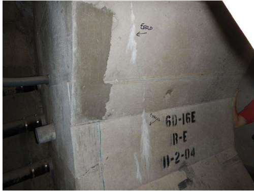
Photo 13 Cracking and efflorescence at the vertical face of the walk through area of the diaphragm at Pier 3D.
