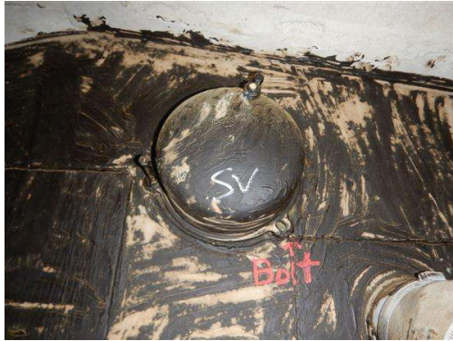
Photo 1 Small void in the PT end cap of T3 tendon and missing cap bolt at Pier 2D.
