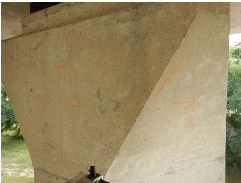
Photo 5 Typical hairline to medium width vertical cracking in the pier cap.
