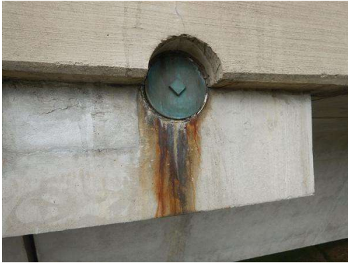
Photo 13 Heavy rust staining and efflorescence on the edge face of the pier end segments.
