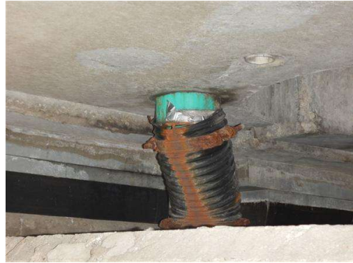
Photo 14 Disconnected drainage pipes and rusted clamps at Pier 4D.
