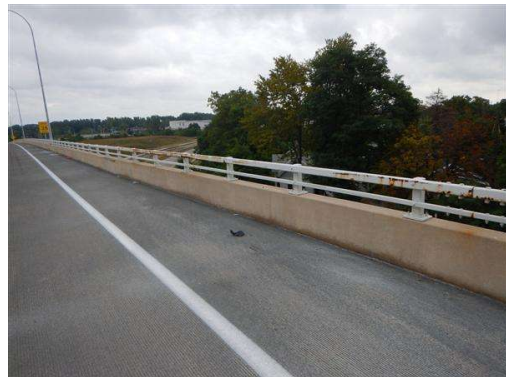
Photo 10 Area of minor deterioration and rust on the steel railing in Span 8D.
