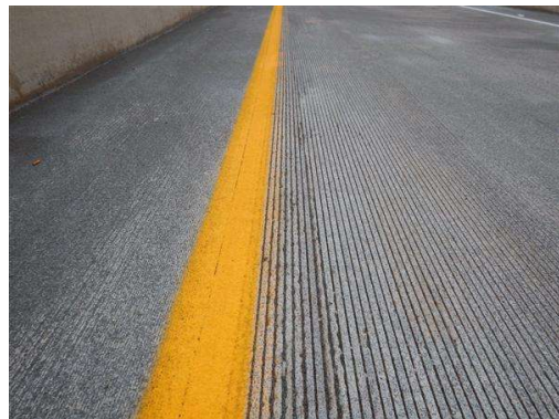
Photo 6 Area of scaling and abrasion in the wearing surface along the east side of the travel lane in Span 9D.
