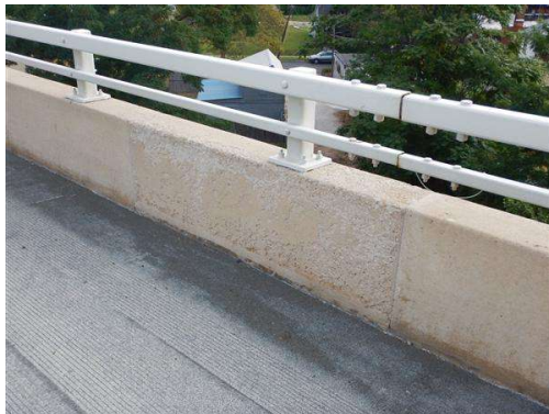
Photo 9 Area of concrete scaling along the vertical face of the east parapet in Span 3D.
