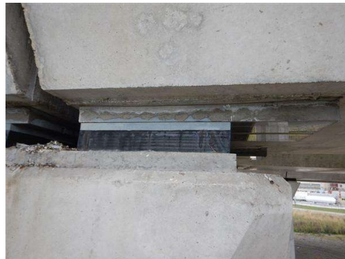
Photo 16 Pier 4D northeast bearing contracted to within 1/4 in. of the edge of the sliding plate.
