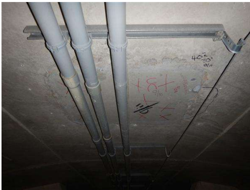
Photo 3 Delaminated concrete and efflorescence in top flange patch located in Span 2D.
