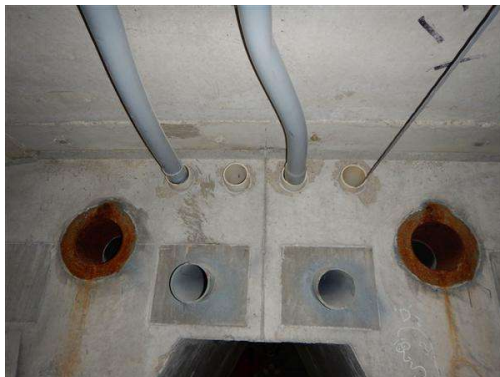
Photo 5 Typical moderate rusting on the future PT ducts located in the diaphragms.
