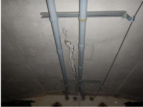
Photo 7 Longitudinal cracking in the top flange/slab concrete with heavy efflorescence.
