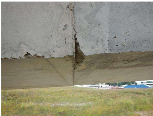
Photo 5 Spalled concrete at segment joint in Span 12D.
