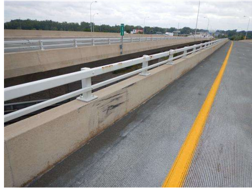
Photo 8 Collision damage/scraping to the west parapet and steel railing in Span 9D.
