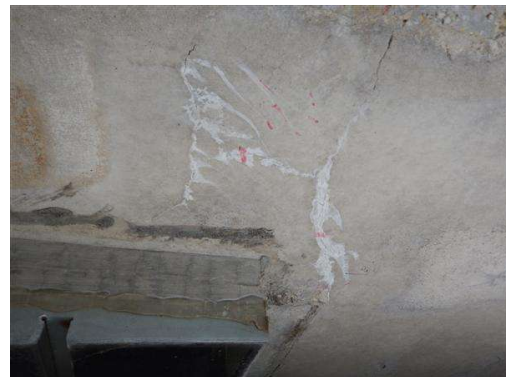
Photo 6 Area of efflorescence in the bottom flange and closure pour near bearing in Span 3D.
