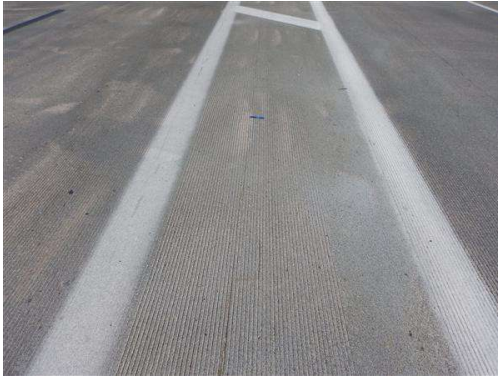
Photo 1 Longitudinal joint with cracking and efflorescent leaching.
