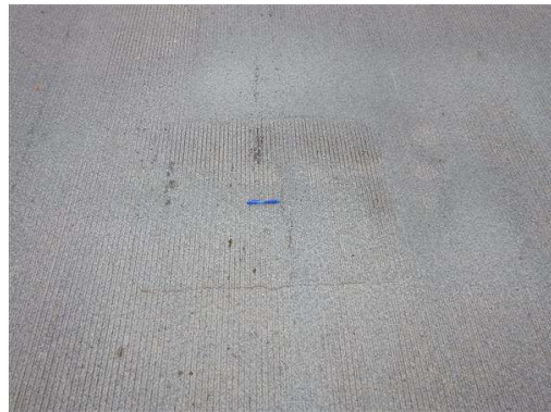
Photo 4 Delaminated patch in the deck/wearing surface with hairline map cracking in the patch in Span 8D.
