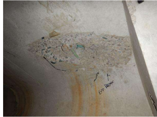
Photo 2 Spalled concrete and exposed reinforcement at a lift hole in Span 10D.
