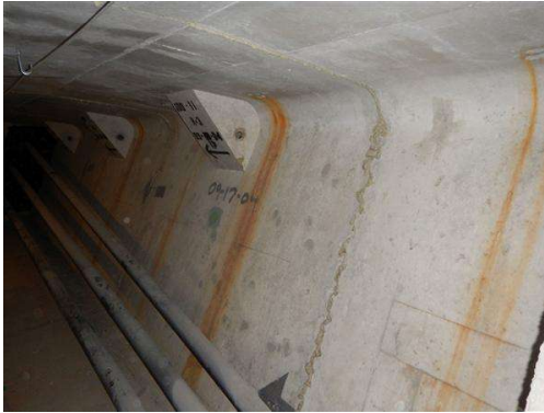
Photo 1 Typical lift hole patches with rust staining leaching from the holes.
