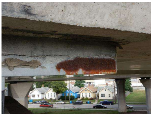
Photo 17 Pier 1D steel sliding plate with an area of rust on the east edge.
