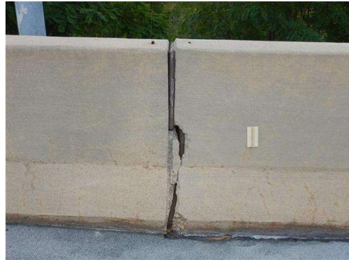
Photo 4 East barrier with vertical displacement/rotation, spalling and cracking of the concrete at the midspan of the approach slab.
