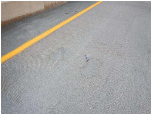
Photo 3 Lift hole patch in the deck/wearing surface with cracks and spalling around the perimeter in Span 8D.
