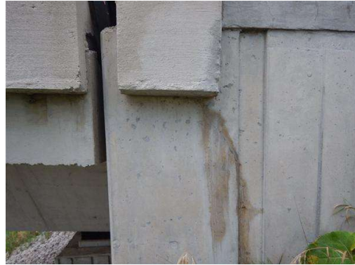
Photo 2 Diagonal cracking with efflorescence on the east end of the Abutment 13D backwall.
