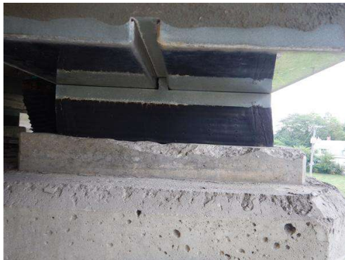
Photo 15 Spall in the east bearing pedestal at Pier 4D and pad leaning toward the west.
