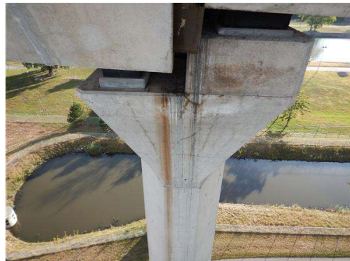
Photo 4 Typical cracking, efflorescence and rust staining on the pier caps
