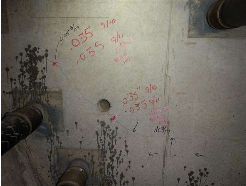
Photo 25 Map cracking on the vertical face of diaphragm at Pier 2SB looking North
