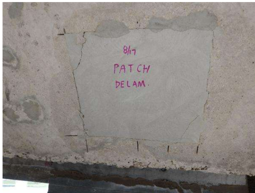
Photo 9 Delaminated concrete patch in the web at Pier 17SB looking West
