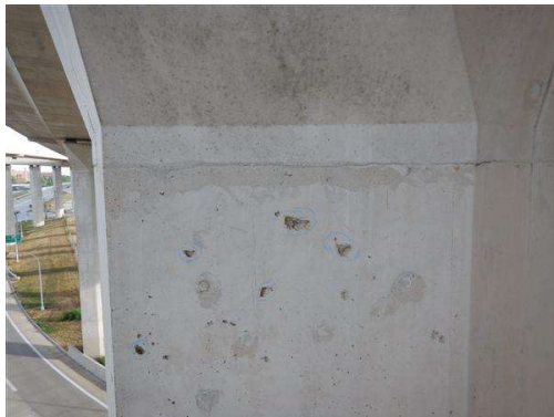
Photo 3 Concrete popouts at Pier 15SB
