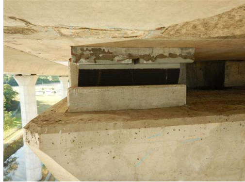
Photo 32 East bearing at Pier 26SB shifted 7.5" North
