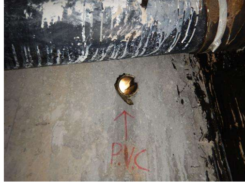
Photo 8 PVC pipe in the web in Span 22SB looking West
