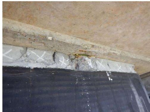
Photo 28 Spalls and delaminated concrete in the East bearing plinth at Pier 9SB
