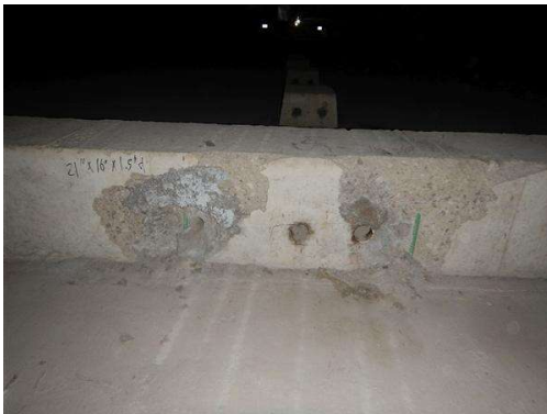
Photo 27 Spall with exposed reinforcement on the North face of bottom strut diaphragm in Span 25SB looking South
