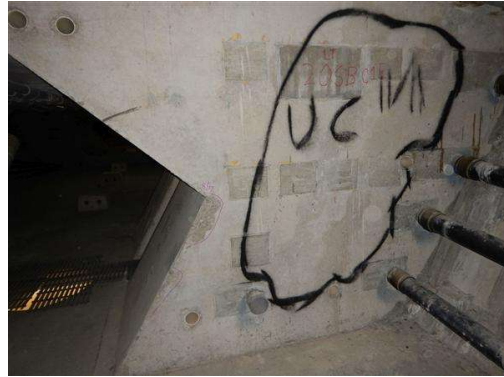
Photo 26 Delaminated concrete area in the vertical face of the diaphragm at Pier 20SB looking South
