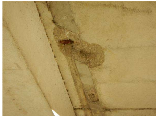
Photo 10 Spall with exposed reinforcement in the cantilever portion of Span 25SB looking East
