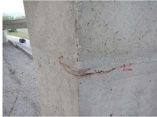
Photo 2 Spall at the construction joint of the column at Pier 13SB
