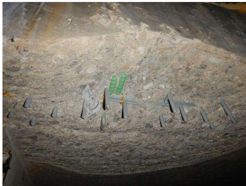
Photo 3 Spall with exposed reinforcement at the expansion joint in Span 8SB looking South
