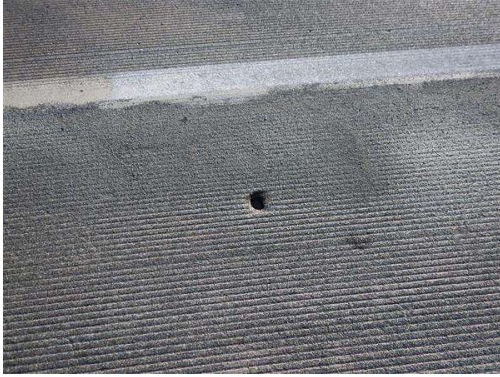
Photo 7 Hole in the deck between Spans 18SB and 19SB
