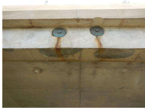
Photo 14 Typical rust staining and efflorescence on the edge face of the end segments
