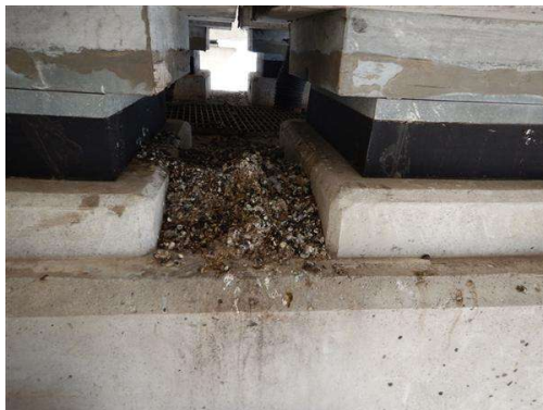
Photo 5 Bird debris on pier cap at Pier 18SB looking West
