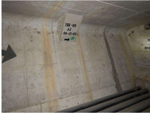
Photo 1 Rust stains from lift holes in Span 7SB
