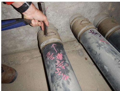
Photo 5 Soft PT duct splices at Pier 7SB looking South
