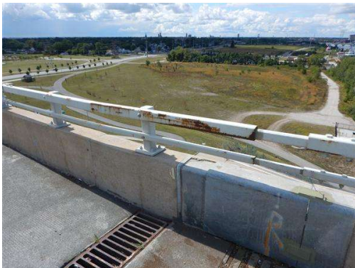
Photo 11 Rust on the steel railing (5' long) in Span 25SB looking West
