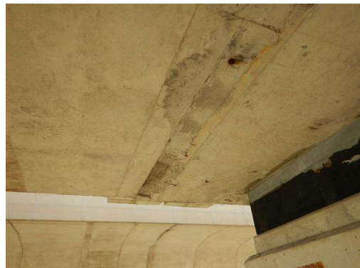
Photo 12 Spall in the bottom flange closure pour between Segments 1 and 2 in Span 24SB
