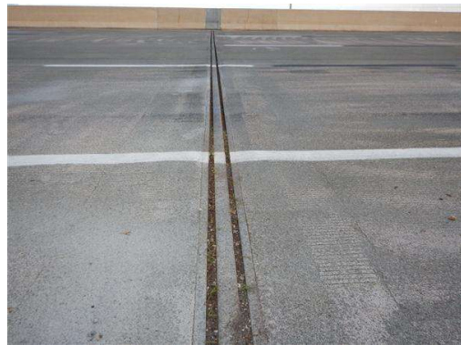
Photo 16 Expansion joint at Pier 24SB filled with debris and growing vegetation looking West
