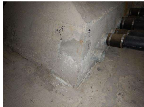
Photo 6 Unsound concrete patches at the base of the deviator wall in Span 9SB looking Southwest
