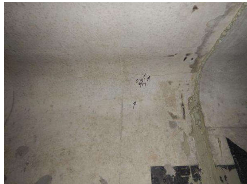
Photo 16 Typical interior upper corner web cracks
