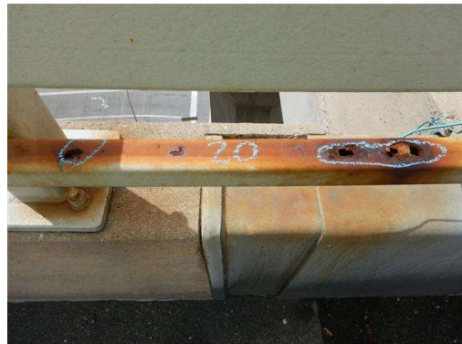
Photo 12 Rust and section loss on the steel railing in Span 5SB looking West
