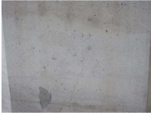
Photo 1 Typical cracking, efflorescence and rust staining on the pier columns
