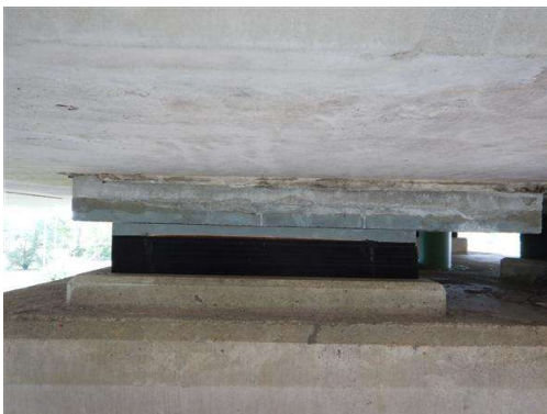
Photo 29 Rust on bearing plate and efflorescence in the plinth of the Southeast bearing East face at Pier 9SB
