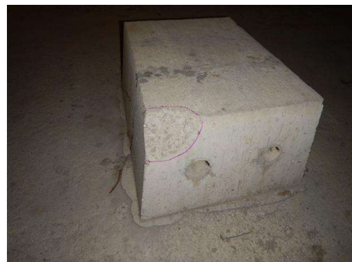
Photo 24 Spall on floor slab PT block in Span 15SB looking North
