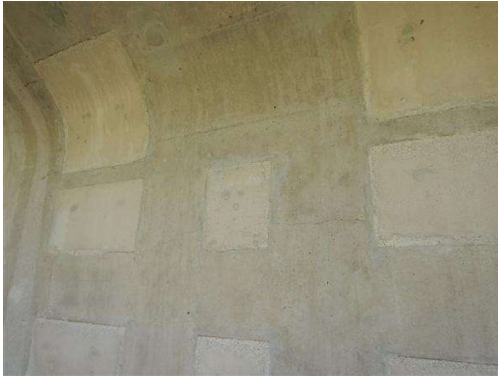
Photo 19 Longitudinal cracks in the West web closure pour in Span 8SB looking East
