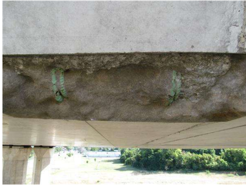
Photo 13 Spall with exposed reinforcement in the bottom flange between Segments 9 and 10 in Span 17SB
