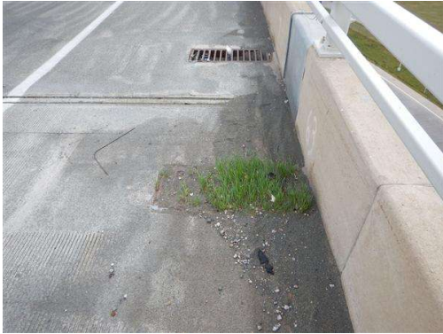
Photo 13 Fully filled scupper with vegetation growing at Pier 20SB
