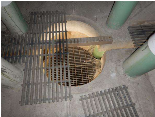
Photo 9 Loose grate at Pier 17SB
