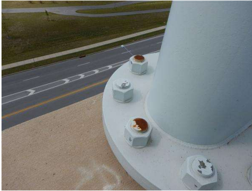
Photo 1 Rusted bolts on the base of the West sign post in Span 23SB looking West
