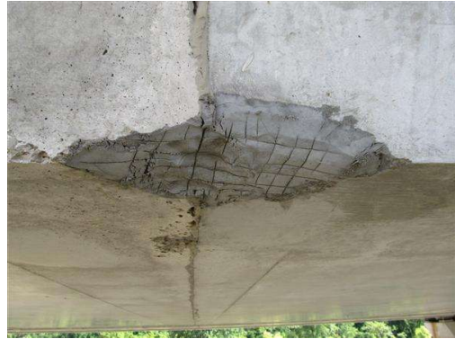
Photo 14 Poor patch on the bottom flange between Segments 9 and 10 on east side of Span 14SB
