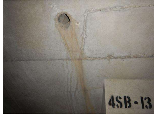
Photo 2 9" deep lift hole unfilled with rust stains in Span 4SB
