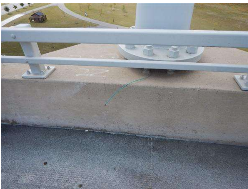
Photo 3 Disconnected grounding wire in Span 23SB
