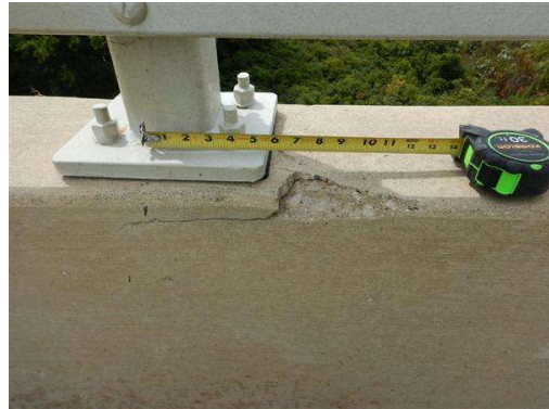
Photo 10 Spall beneath the steel railing in Span 5SB
