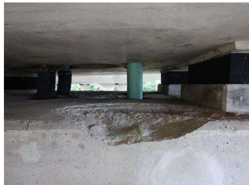
Photo 6 Spall (36"x48"x5") with exposed reinforcement at Pier 11SB
