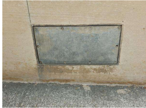
Photo 2 Missing and loose screws in the electrical panel in Span 5SB
