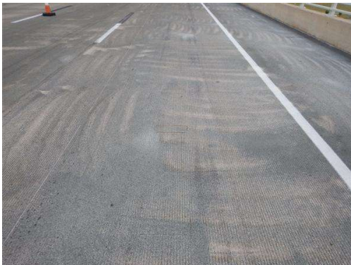
Photo 3 Typical concrete patches in the traffic lane between Spans 24SB and 25SB
