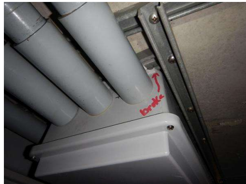
Photo 10 Loose junction box and broken mounting tab in Span 25SB looking North
