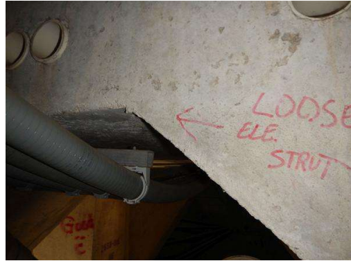
Photo 8 Loose electrical conduit strut in Span 25SB looking North
