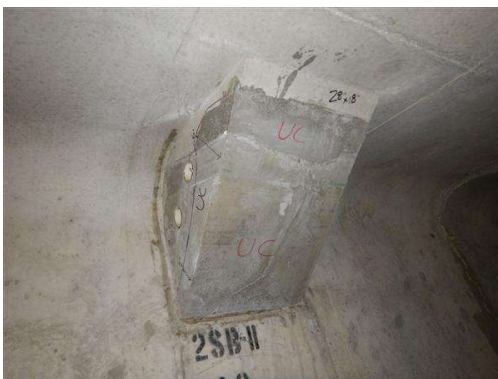
Photo 23 Delaminated concrete patches on future PT block in Span 2SB looking West
