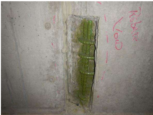
Photo 21 5" deep concrete void with exposed reinforcement in Span 21SB looking West
