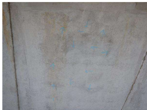
Photo 18 Typical hairline map cracking on the exterior webs along the length of the bridge
