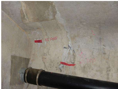
Photo 15 Cracks with efflorescence in the web to top slab corner in Span 8SB looking East
