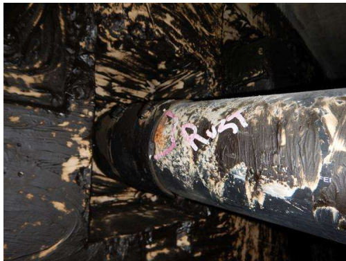
Photo 3 Rust on PT duct at Pier 3SB looking North
