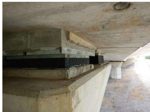
Photo 30 Spall in the West bearing pedestal at Pier 3SB
