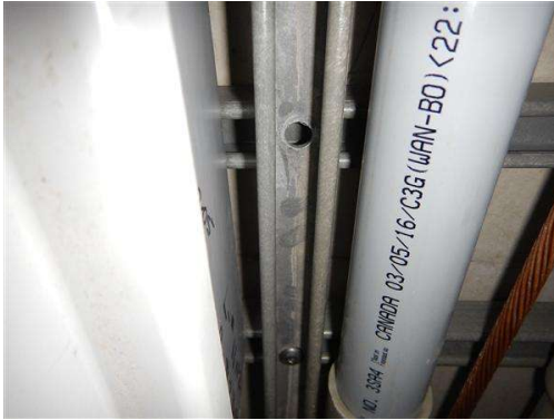
Photo 7 Missing bolt from electrical conduit strut in Span 13SB looking North
