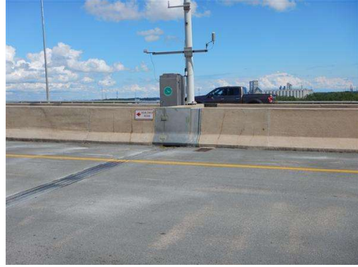
Photo 8 Typical vertical cracking with rust stains along the East parapet looking East
