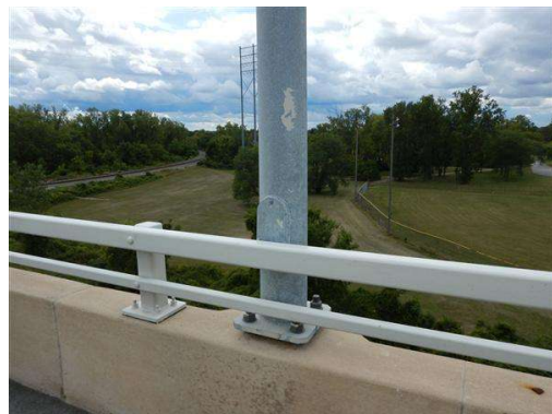
Photo 4 Paint or coating failure on electrical pole on west parapet in Span 8SB looking West
