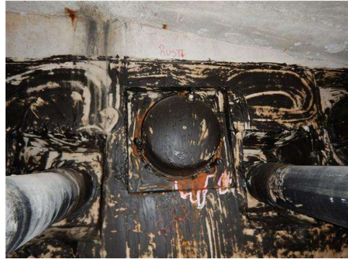
Photo 2 Voids and rust around the perimeter of the PT anchor cap at Pier 6SB looking South
