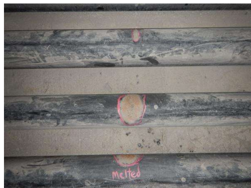
Photo 6 Plastic on PT duct appeared melted in Span 23SB
