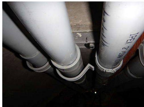
Photo 6 Broken electrical conduit bracket in Span 8SB looking South
