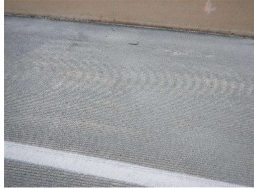
Photo 2 Transverse cracks in the shoulder between Spans 22SB and 23SB
