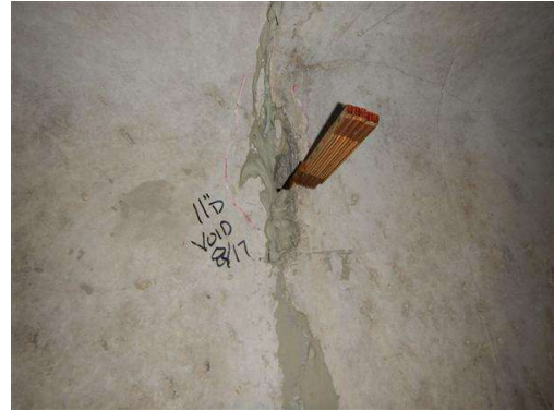
Photo 20 11" deep void in the interior construction joint in Span 14SB
