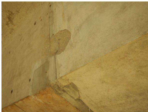
Photo 11 Spall in the East web between Segments 1 and 2 in Span 25SB
