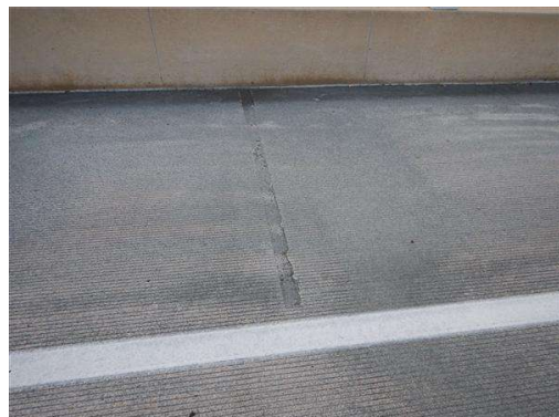
Photo 6 0.25" depression in the shoulder between Spans 24SB and 25SB
