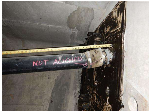
Photo 4 PT cable T3 not aligned at Pier 18SB looking East
