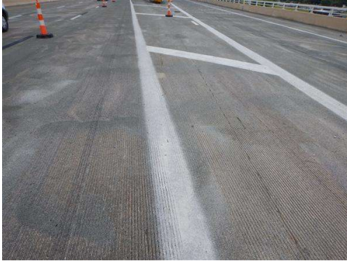
Photo 1 Longitudinal cracks in the longitudinal joint between Spans 21SB and 22SB looking South
