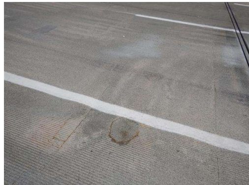
Photo 4 Concrete patch with spalls and discoloration around perimeter between Spans 24SB and 25SB
