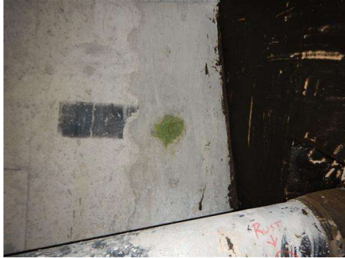
Photo 7 Exposed reinforcement in the closure pour joint in Span 7SB looking West
