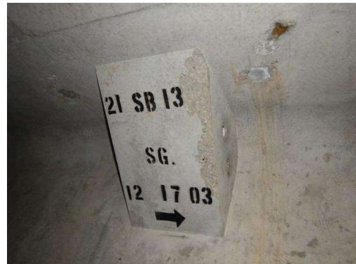
Photo 22 Typical spalls in the future PT blocks
