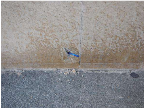
Photo 9 Spall in the parapet in Span 24SB
