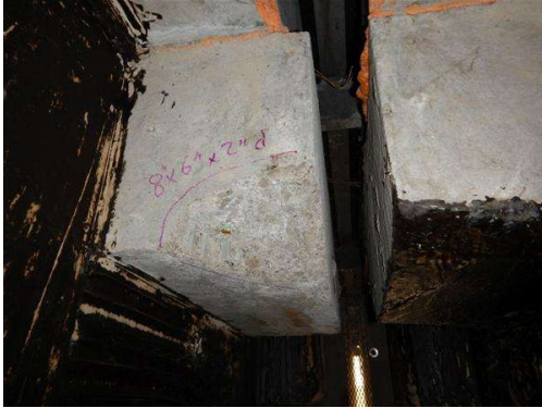
Photo 25 Spall with exposed reinforcement in the PT concrete end block in Span 15NB looking West
