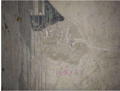
Photo 7 Spall (16"x16"x2") in web in Span 19NB looking West
