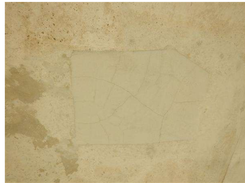
Photo 10 Concrete patch with map cracks in the bottom flange of Spans 21NB and 22NB
