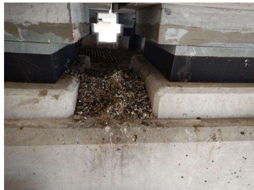
Photo 6 Bird debris on the cap at Pier 18NB looking West
