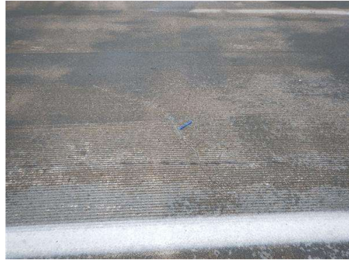
Photo 2 Moderate map cracks in the approach slab looking West
