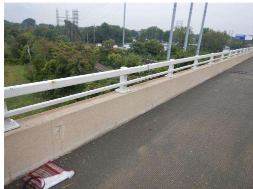
Photo 12 Typical vertical and horizontal cracks in the East parapet of Span 5NB looking East
