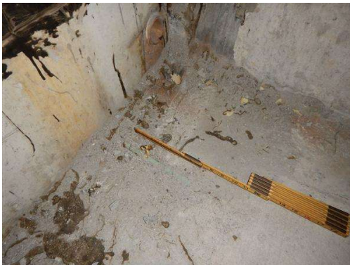
Photo 21 Exposed reinforcement on the floor of Span 18NB looking Northeast
