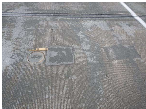
Photo 6 Depressed concrete patch with discoloration around perimeter between Spans 1NB and 2NB
