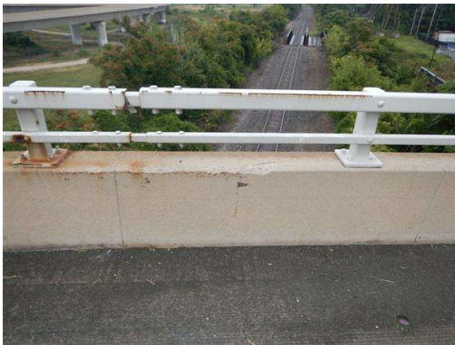
Photo 15 Minor rust and section loss in the steel railing in Span 5NB looking East
