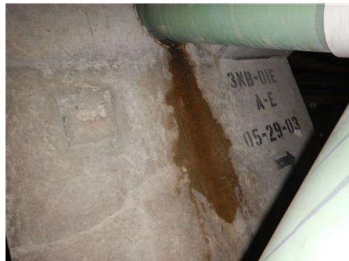
Photo 18 Interior drainage pipe with rust staining at Pier 3NB
