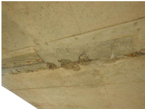
Photo 9 Spall (4'x 8"x1") with 0.01" crack in the bottom flange of Spans 21 NB and 22NB
