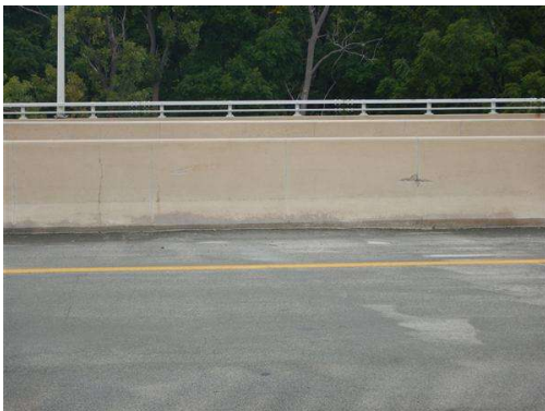
Photo 11 Typical vertical cracks and spall in West parapet of Span 4NB looking West
