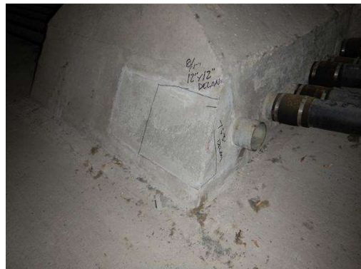
Photo 18 Delamination (12"x12") in the deviator wall of Span 5NB looking Southwest
