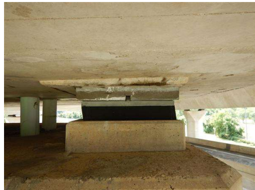
Photo 28 Efflorescence on the plinth and bearing plate at Pier 11NB East bearing
