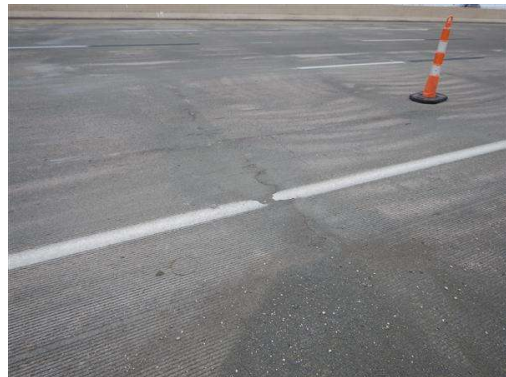
Photo 10 Deck surface worn out between Spans 14NB and 15NB looking West
