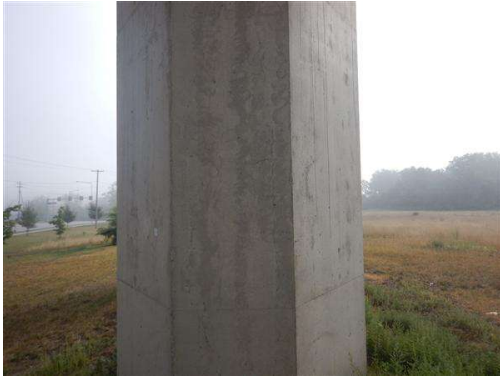
Photo 1 Vertical cracks in the column at Pier 19NB
