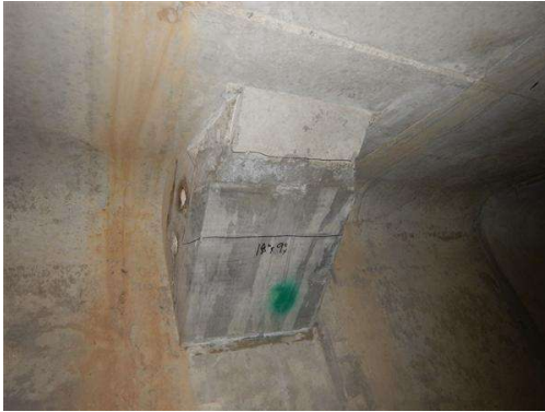
Photo 19 Delamination (18"x18") and spall (6"x6"x1") in web exterior PT block in Span 10NB looking East
