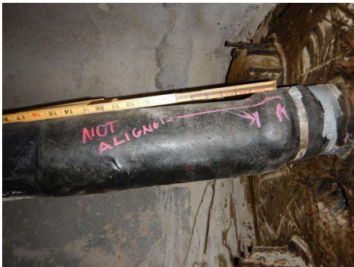
Photo 3 PT duct pipe not aligned at Pier 19NB looking East
