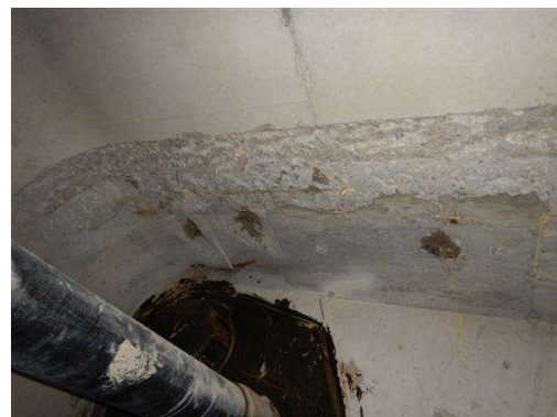
Photo 6 Full width spall in top flange in Span 17NB looking South
