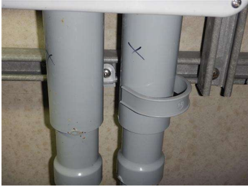
Photo 1 Broken electrical conduit bracket at Pier 1NB
