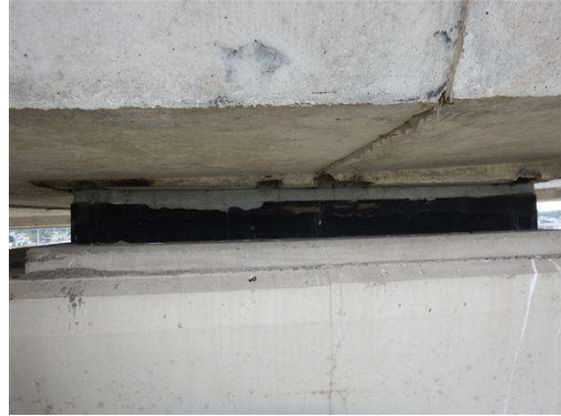
Photo 26 Four (4) spalls in the plinth at Pier 24NB
