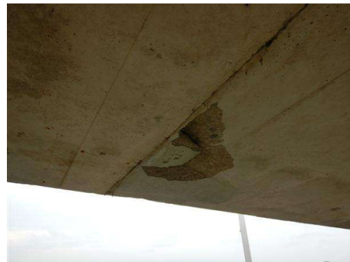
Photo 12 Spall (20"x15"x2") with exposed reinforcement in bottom flange of Spans 24NB and 25NB
