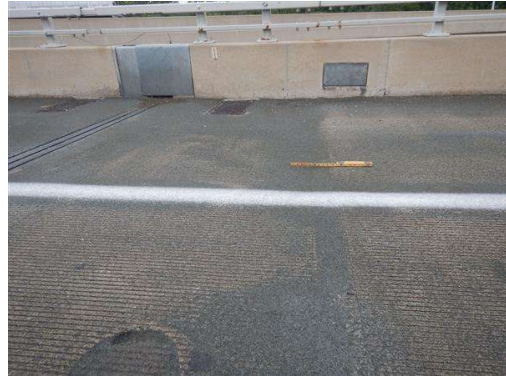
Photo 8 Deck discontinuity between segments and not smooth riding surface between Spans 8NB and 9NB
