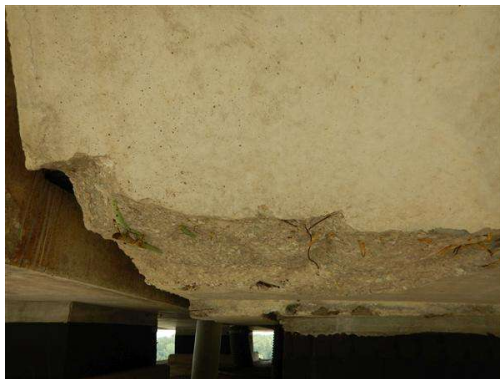
Photo 11 Spall (3'x28"x4") with exposed reinforcement in the bottom flange of Spans 22NB and 23NB
