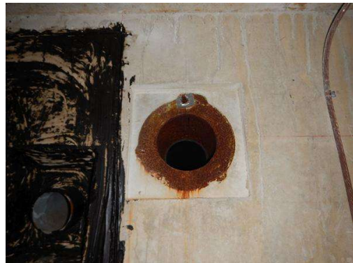
Photo 4 Heavy rust on the future PT ducts at Pier 3NB looking North
