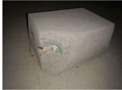
Photo 20 Spall with exposed reinforcement on future PT block in Span 21NB looking East
