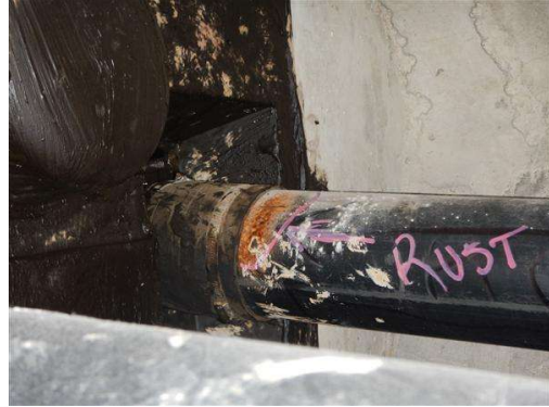
Photo 2 PT clamp rust at Pier 5NB looking North
