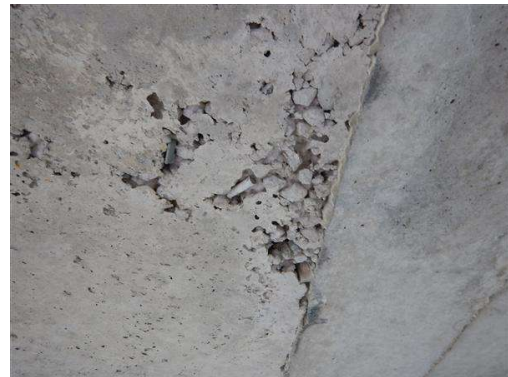
Photo 22 Honeycombed concrete in the bottom flange of Spans 6NB and 7NB
