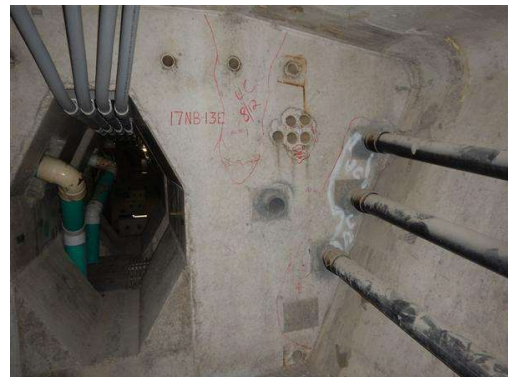
Photo 24 Delaminated concrete patch (12"x39") and map cracking in diaphragm in Span 17NB looking North
