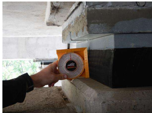
Photo 30 East bearing bulging out North at Pier 11NB looking West
