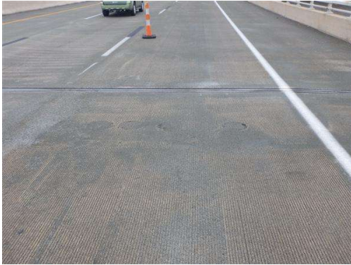
Photo 7 Lift hole patches with spall between Spans 8NB and 9NB
