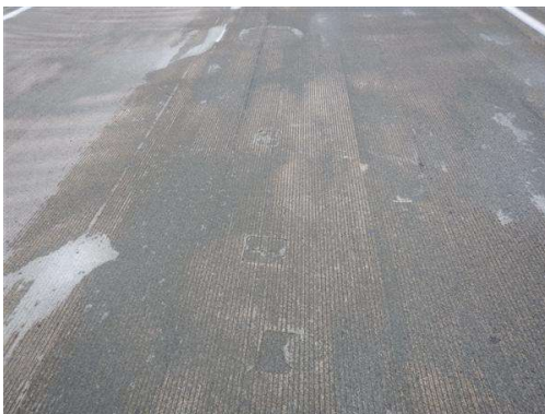
Photo 5 Concrete patches with map cracking around the perimeter between Spans 1NB and 2NB
