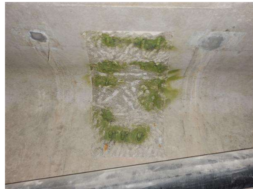
Photo 4 Temporary jacking block removed exposing reinforcement and no patch in Span 15NB looking East
