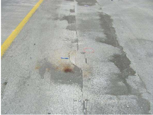
Photo 1 Typical transverse closure pour joint cracking with efflorescence
