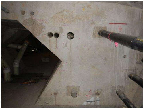
Photo 23 Map cracking (0.005" to 0.030") in the diaphragm in Span 10NB looking North
