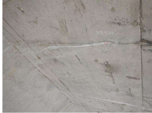
Photo 2 Bottom of the deck slab closure pour transverse cracks with heavy efflorescence looking North
