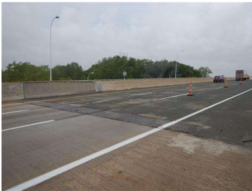
Photo 3 Growing vegetation on the East side of the relief joint looking West
