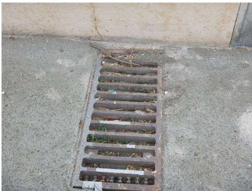
Photo 17 Scuppers fully clogged with debris in Span 22NB
