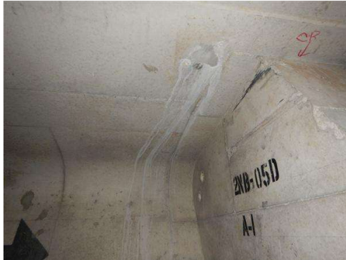
Photo 1 Efflorescence leaching from lift holes at 2NB looking West
