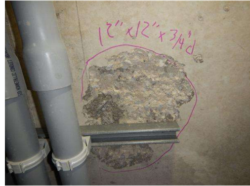
Photo 8 Spall (12"x12"x0.75") in top flange of Span 22NB
