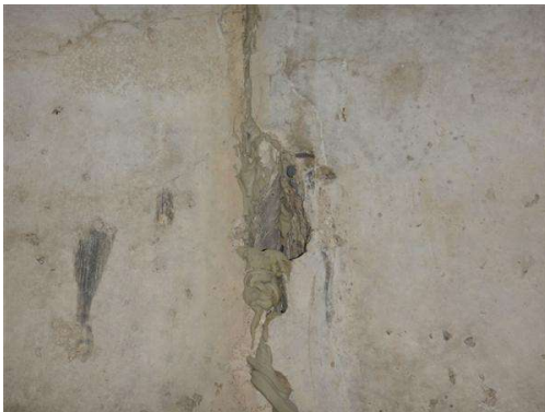
Photo 15 10 inch deep void in web of Span 12NB looking East
