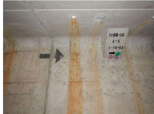
Photo 2 Rust stains at lift holes at 10NB looking West
