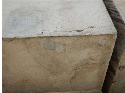
Photo 14 Longitudinal crack with concrete popout in the web at Pier 23NB
