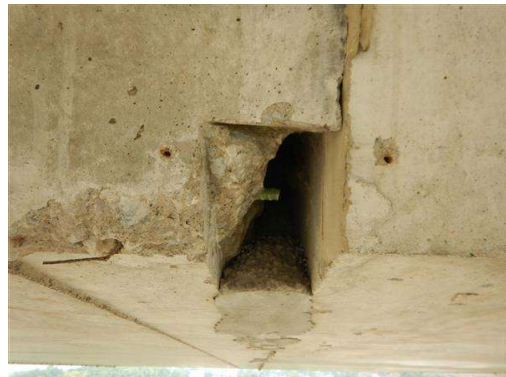
Photo 16 Void (15"x3.5"x6") in the bottom flange of Spans 21 NB and 22NB
