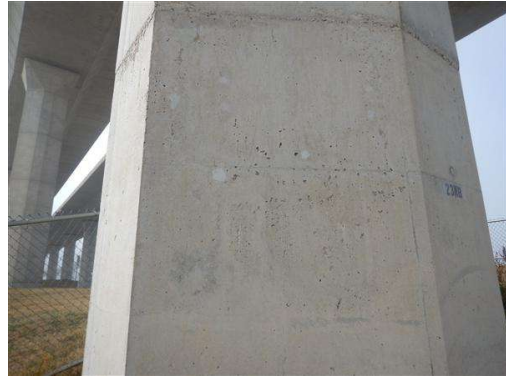
Photo 2 Typical honeycombing on a majority of columns
