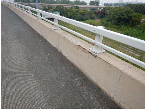
Photo 13 Collision damage (2.5' long) on East parapet of Span 3NB looking Northeast
