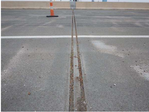
Photo 19 Expansion joint at Pier 20NB filled with debris and growing vegetation looking West
