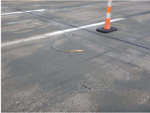
Photo 1 Concrete spalls of varying sizes in approach slab looking West
