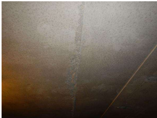
Photo 3 Spall along the construction joint in top flange in Span 3NB looking North
