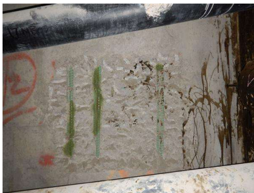
Photo 5 Spall (3'x3'x3") in web exposing reinforcement in Span 17NB looking East
