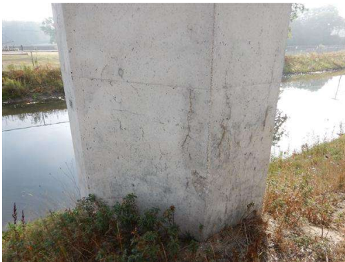
Photo 3 Spall and map cracking at Pier 25NB
