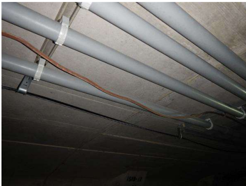
Photo 3 Ground cable is hanging at Pier 15NB
