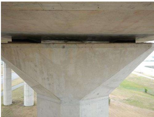
Photo 5 Hairline to moderate map cracks on the South face of Pier 21NB
