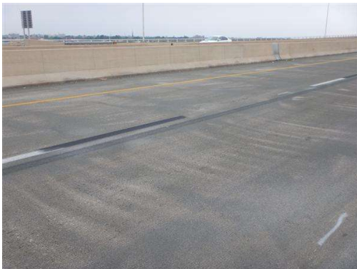
Photo 9 Scaling of the deck surface between Spans 19NB and 20NB looking West
