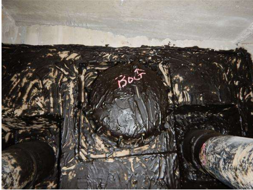
Photo 1 Bolt missing and rust on tendon duct at PT anchor cap at Pier 3NB looking North
