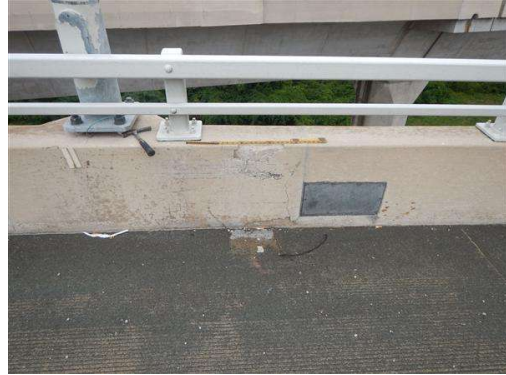
Photo 14 Delaminated/spalled concrete (26"x2.5") in Span 9NB of East parapet looking East
