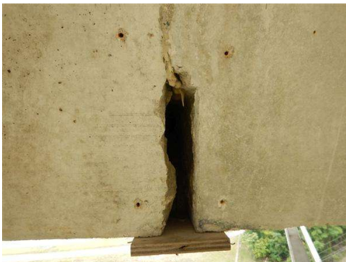
Photo 17 Void (19" deep) at the construction joint between Spans 23NB and 24NB
