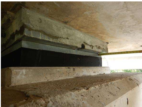
Photo 29 East bearing shifted 3" South at Pier 9NB looking East
