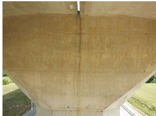
Photo 4 Typical hairline to moderate cracking with rust staining or efflorescence on pier caps
