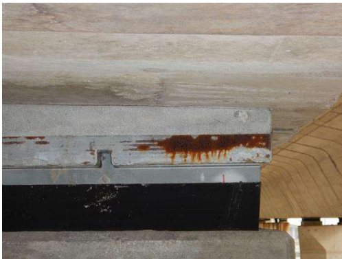
Photo 27 Rust on the East bearing plate at Pier 14NB
