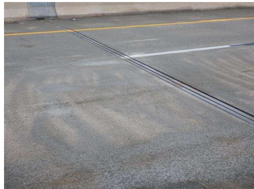
Photo 4 Transverse cracks at the expansion joint between Spans 8NB and 9NB looking West
