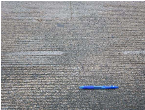
Photo 3 Transverse cracks at the construction joint between Spans 1NB and 2NB
