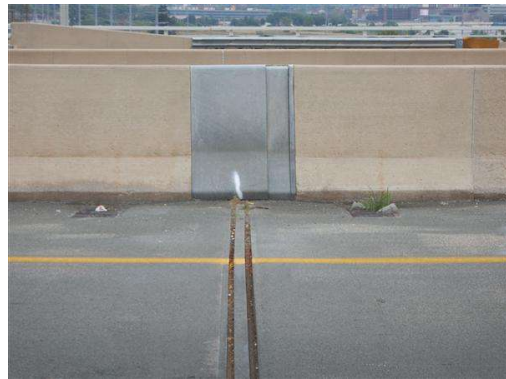
Photo 16 Vegetation growing out of scuppers in Span 19NB looking West
