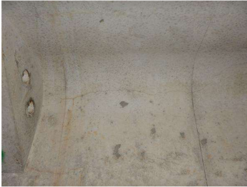
Photo 13 Longitudinal cracks in web in Span 9NB looking East
