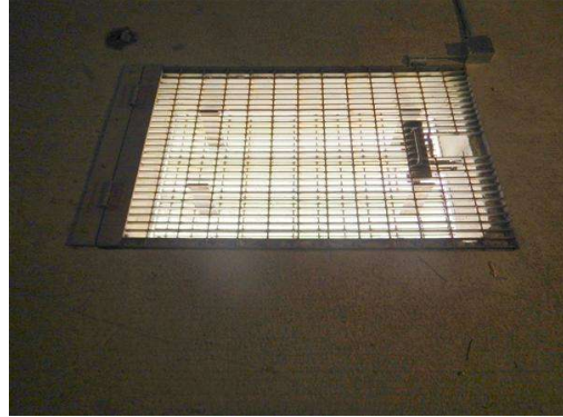
Photo 2 Access hatch not tied down at Pier 3NB
