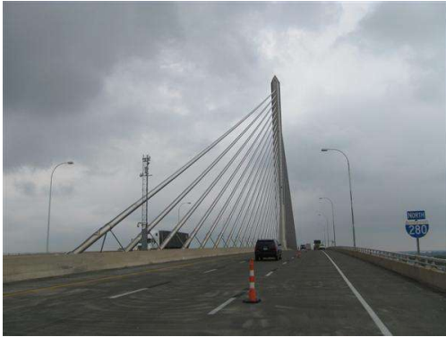
Photo 1 Faded I-280 North sign
