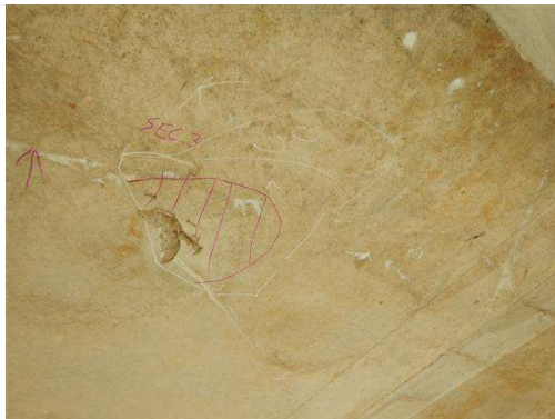
Photo 15 Delaminated concrete patch (12"x12") in the exterior bottom flange of Span 27NB
