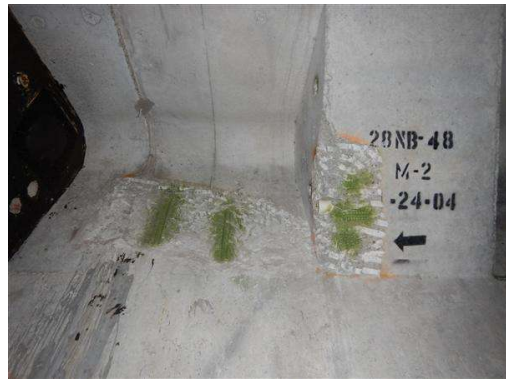
Photo 28 Typical spall with exposed reinforcement in the future PT blocks in webs
