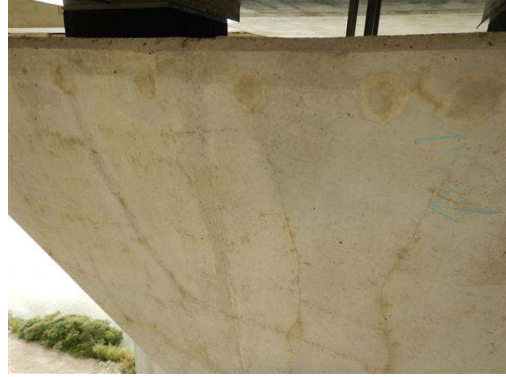
Photo 2 Typical cracking and rust stains in the Southbound pier caps
