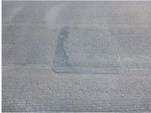
Photo 7 Concrete patch (4'x2') in the traffic lane in Span 28SB
