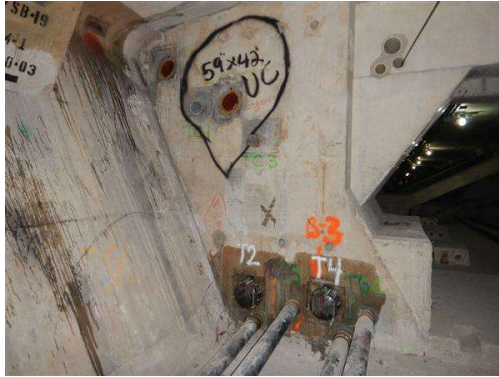
Photo 55 Delaminated concrete area in the vertical face of the diaphragm in Span 27SB
