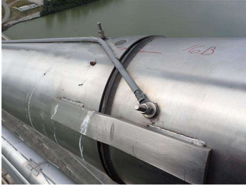
Photo 25 0.75" gap between the original caulk and the end of the upper sleeve. Full circumference gap between upper sleeve and cradle sheath on Cable Stay 16B upper sleeve
