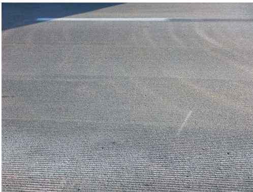
Photo 5 Transverse cracks in the traffic lane in Span 28SB
