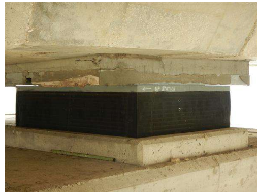
Photo 58 Gap between load plate and sole plate on West bearing at Pier 29NB
