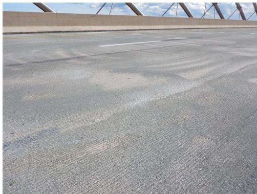
Photo 11 Scaling in the wearing surface of Span 27SB
