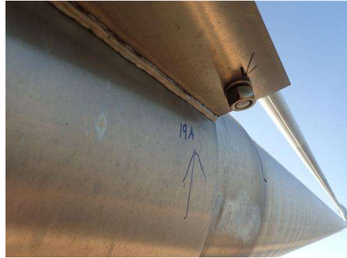
Photo 20 South bolt on the West cable damper clamp loose at Cable Stay 19A
