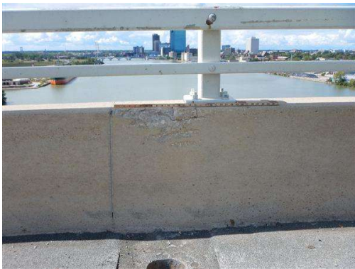
Photo 21 Spall underneath the steel railing in Span 27SB looking West
