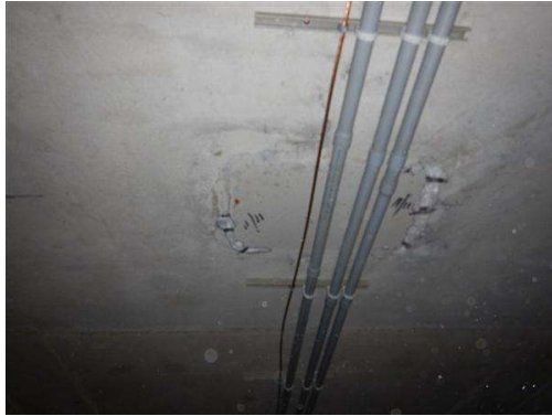
Photo 13 Construction access hole patch with cracks and leaching efflorescence in Span 27NB
