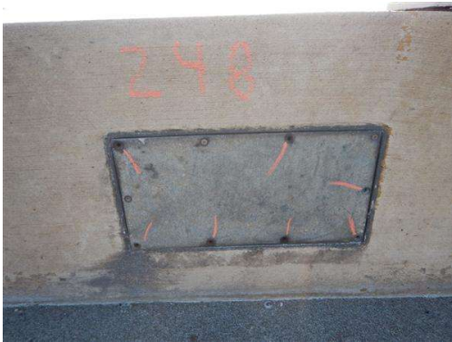
Photo 3 Missing screws in the electrical junction box on the East parapet in Span 29NB
