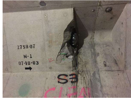
Photo 50 Spalls with exposed reinforcement in the diaphragm block in Span 27SB
