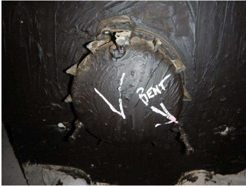
Photo 1 Void in the PT anchor cap at Pier 27NB
