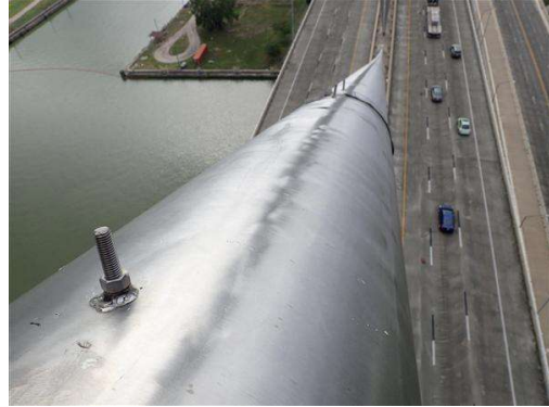
Photo 26 No ground wire present on Cable Stay 9B upper sleeve
