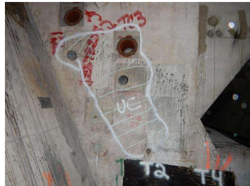
Photo 54 Delaminated concrete area in the vertical face of diaphragm at Pier 27NB
