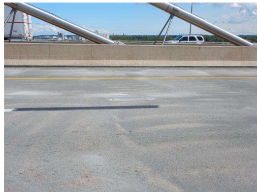
Photo 6 Lift hole patches with leaching efflorescence around perimeter in Span 27SB
