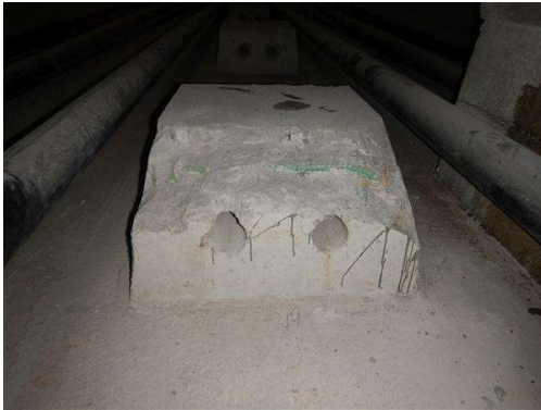
Photo 51 Typical spall with exposed reinforcement in the temporary PT blocks on bottom flange/slab along the length of the bridge
