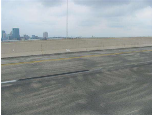
Photo 13 Vertical cracks in the West parapet in the Span 28NB looking West
