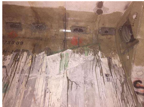
Photo 34 Concrete spall (36"x12"x2") with exposed reinforcement in the web of Span 27SB
