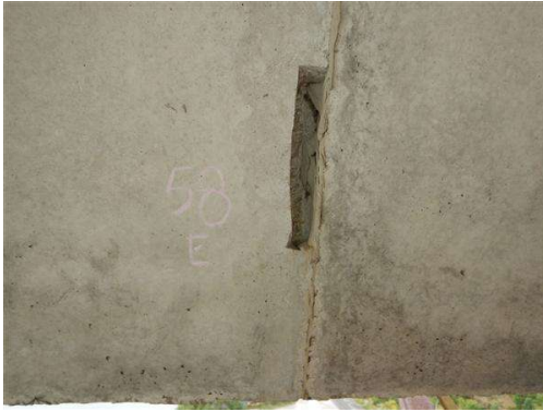
Photo 49 Cutout (3" deep) in the exterior East web between Segments 57 and 58, in Span 28SB looking West
