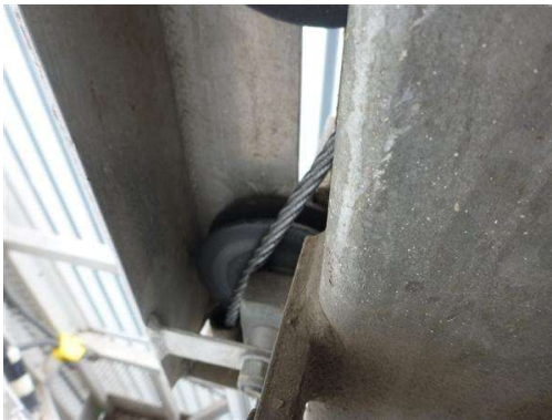
Photo 15 Southeast lift wire rope off sheave
