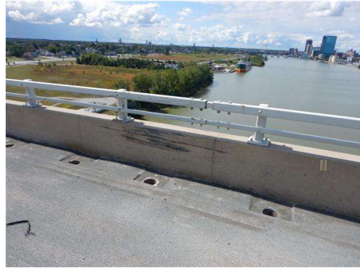
Photo 20 Collision damage to the West parapet in Span 27SB
