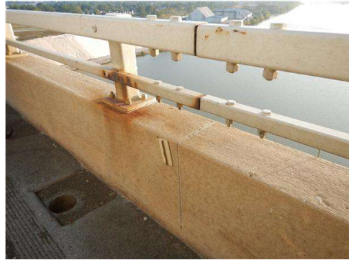
Photo 2 Broken or missing reflectors along the length of the bridge
