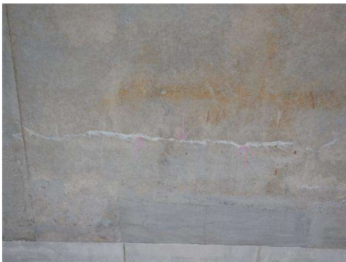
Photo 23 Longitudinal cracks with leaching efflorescence in the exterior bottom flange/slab in Span 27NB
