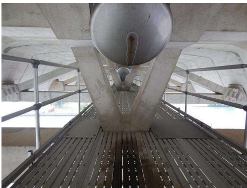
Photo 17 Leaching rust stains from stainless steel sheath at the bottom of deck Stay Cable Anchor 2A
