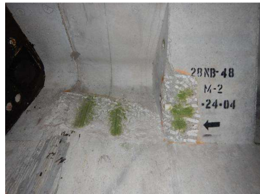
Photo 6 Spalls with exposed reinforcement in the web in Span 28NB looking East
