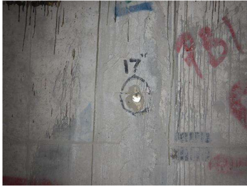
Photo 31 Unfilled hole in web of Span 28SB
