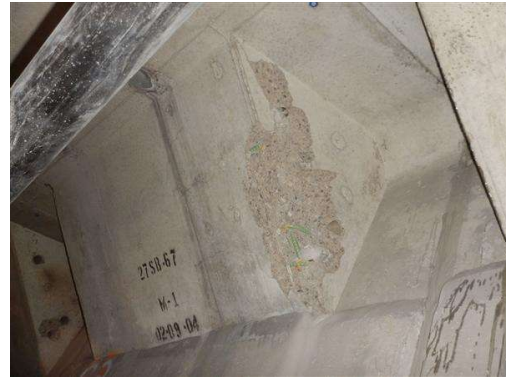
Photo 52 Typical cracks with exposed reinforcement in corbels along the length of the bridge
