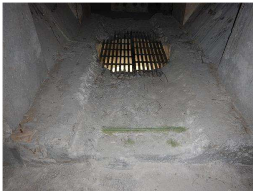
Photo 5 Exposed reinforcement on the bottom flange/slab in Span 29NB looking South
