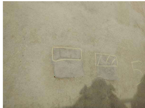
Photo 40 Delaminated patch (8"x4") in the exterior East web of Span 29SB
