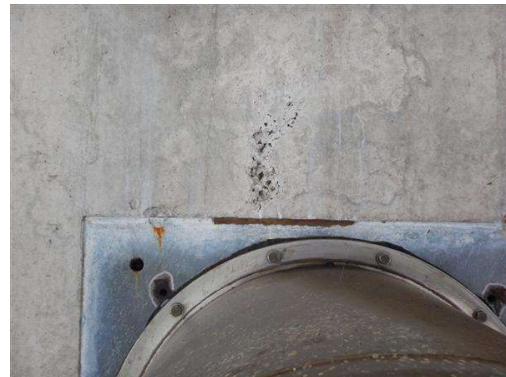
Photo 16 Honeycombed concrete on the top (North face) of deck Stay Cable Anchor 4A
