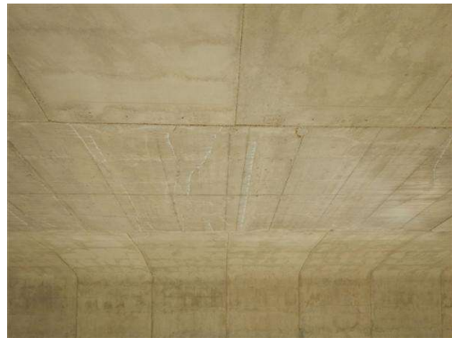
Photo 4 Bottom of the deck slab closure pour with transverse cracks and efflorescence in Segments 5 through 13 in Span 29SB
