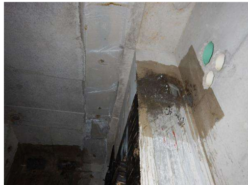
Photo 10 Delaminated patch with leaching efflorescence in Span 29NB looking West
