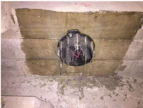
Photo 5 Voids in the PT anchor cap at Pier 27SB
