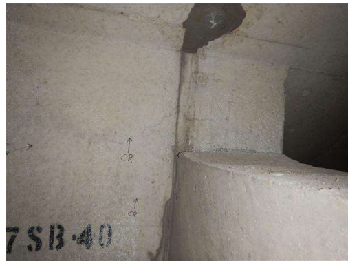
Photo 46 Typical cracks on the diaphragm blocks along the length of the bridge
