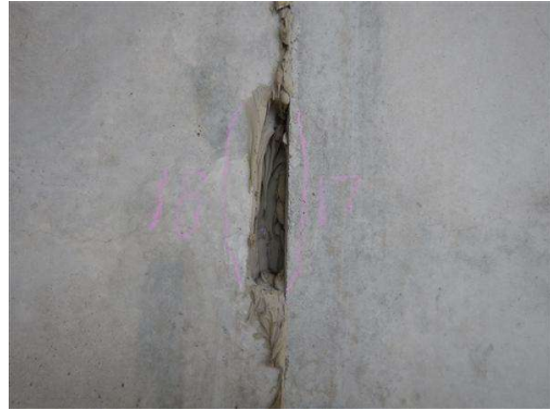
Photo 26 Void (4" deep) between Segments 17 and 18 of Span 28NB
