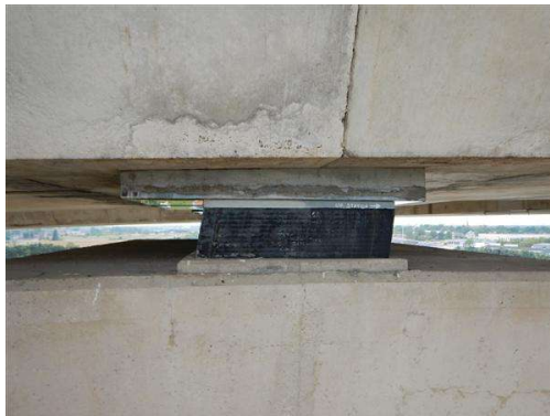
Photo 57 East bearing at Pier 27NB rotated 10° to the North
