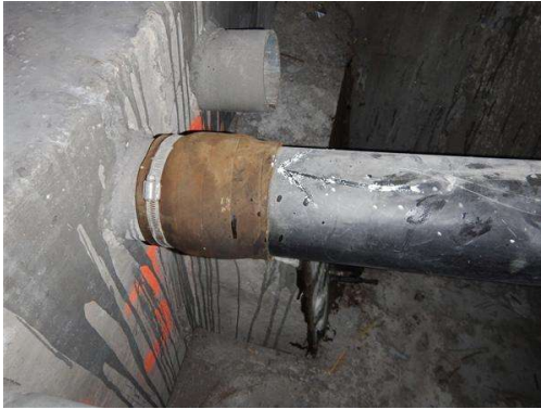
Photo 7 Missing PT clamp at Pier 27NB looking West
