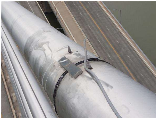
Photo 27 Ground cable disconnected from the lower bolt on the main sheath Cable Stay 20B upper sleeve
