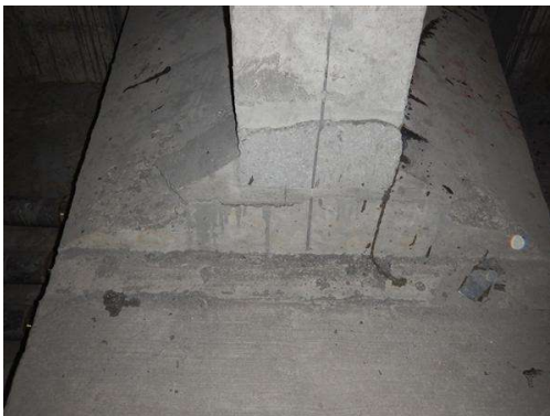
Photo 11 Spalls on the deviator wall at Pier 27NB looking West
