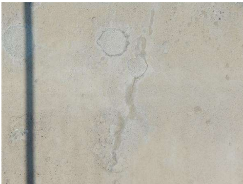
Photo 31 Multiple round patches up to 2" diameter with full perimeter cracking up to .03125" in width with discoloration on the Upper Pylon East face near Cable Stay 9
