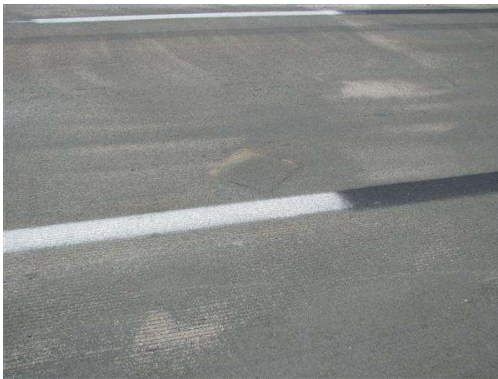
Photo 3 Concrete patch with cracks and discoloration around perimeter in Span 27NB
