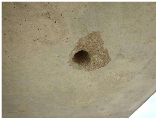
Photo 17 Spall (6"x6"x0.5") at the core hole in Segment 16 of Span 29NB
