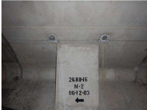
Photo 1 Leaching efflorescence from lift holes in Span 26NB
