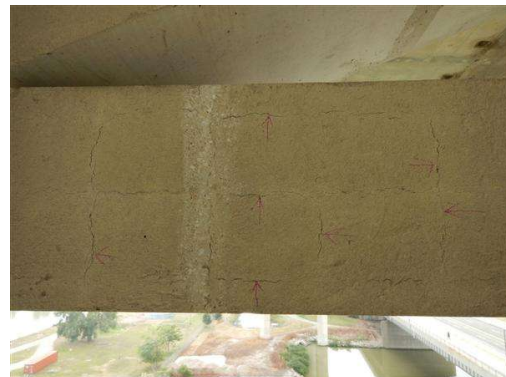
Photo 18 Horizontal and vertical cracks in the lower right strut at Stay Cable Anchor 4B between Segments 53-55 in Span 27NB
