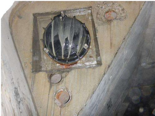
Photo 3 Rusted PT base plate in Span 28SB
