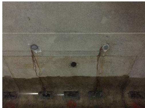
Photo 30 Leaching efflorescence from lift holes in Span 27SB
