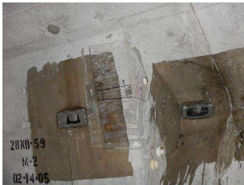
Photo 29 Delaminated patch on future PT block at 28NB looking West
