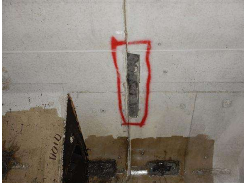
Photo 25 Concrete cutout (2.5" deep) in the top flange/slab at Pier 28NB looking West
