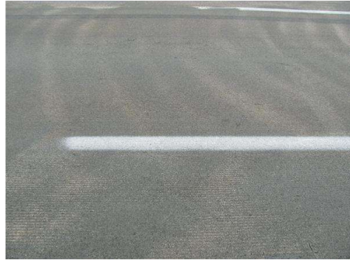
Photo 2 Transverse cracks in the deck in Span 28NB
