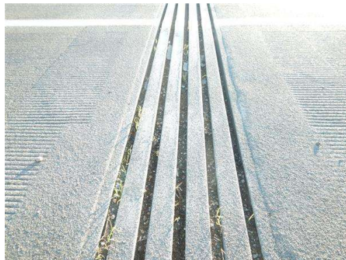
Photo 30 Expansion joint at Pier 29SB filled with debris and growing vegetation
