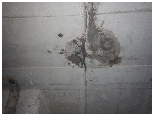
Photo 35 Delaminated/unsound patch and spalls in the top flange/slab in Span 28SB
