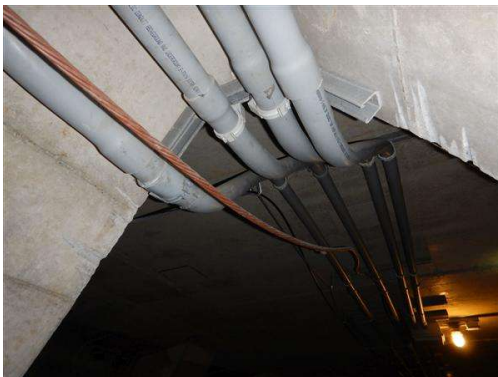
Photo 5 Ground wire not attached to the brackets in Span 26NB
