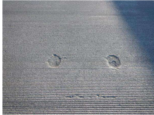
Photo 8 Spalls (7"x5"x0.75") in Span 28SB
