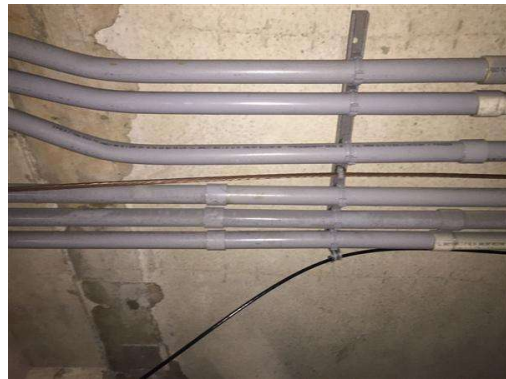
Photo 10 Broken electrical conduit clamp in Span 26SB
