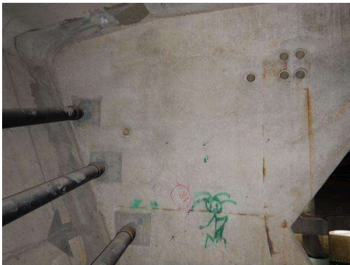
Photo 53 Map cracking on the vertical face of diaphragm at Pier 26NB
