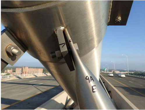
Photo 19 Gap (0.25") between cable clamp and East damper support leg at Cable Stay 9A
