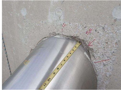
Photo 30 1.5"x1" edge spall around the stay cable from 12 to 2 o'clock on the Upper Pylon South face at Cable Stay 12
