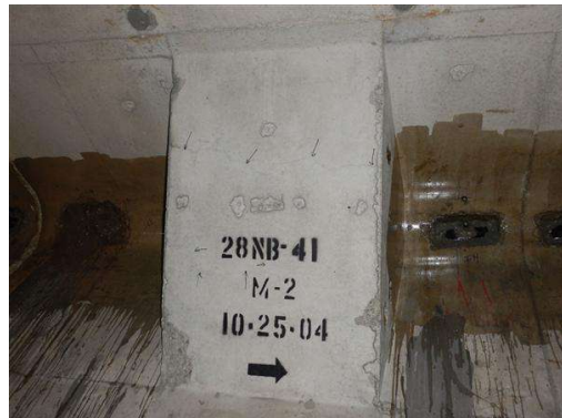
Photo 22 Typical cracks on future PT blocks along the length of the bridge looking West
