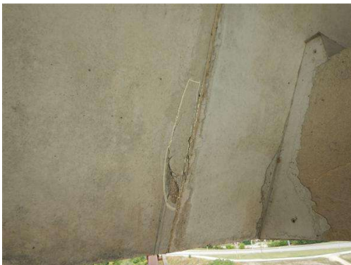
Photo 41 Spall (27"x5"x0.5") in the exterior East web of Span 28SB looking West
