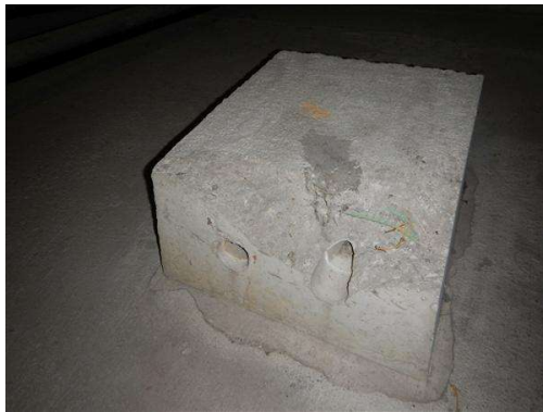
Photo 27 Spalls with exposed reinforcement in future PT block on the bottom flange/slab of Span 29NB looking South
