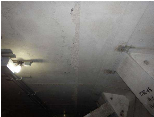
Photo 9 Typical spalls in the top flange/slab looking North
