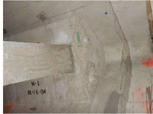
Photo 38 Typical spalls with exposed reinforcement in the corner blocks
