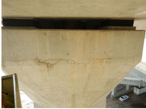
Photo 1 Typical cracking and rust stains in the Northbound pier caps
