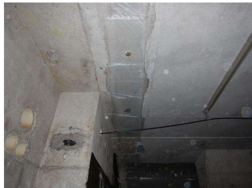
Photo 36 Closure pour with cracks and efflorescence in Span 28SB
