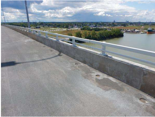
Photo 19 Vertical cracks in newly installed West parapet sections in Span 27SB
