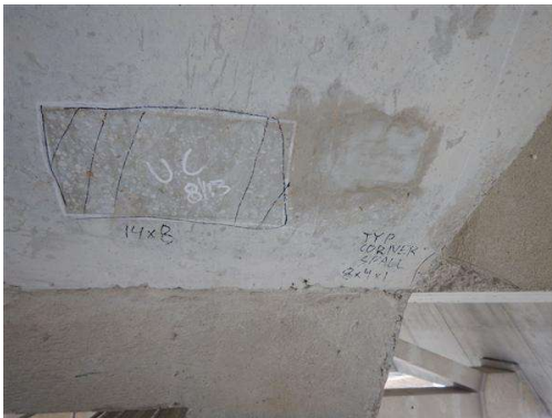
Photo 15 Delaminated/unsound concrete patch on the bottom (North face) of Stay Cable Anchor 8A
