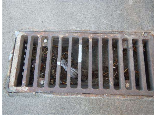
Photo 26 Scupper filled with debris at Pier 30NB
