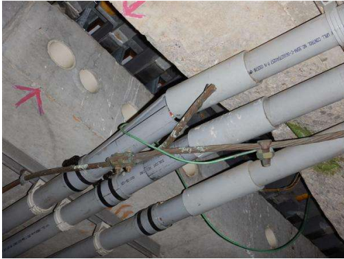
Photo 7 Separated electrical conduit at Pier 29NB
