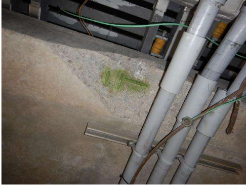
Photo 7 Spalls with exposed reinforcement at expansion joint at Pier 29NB looking South
