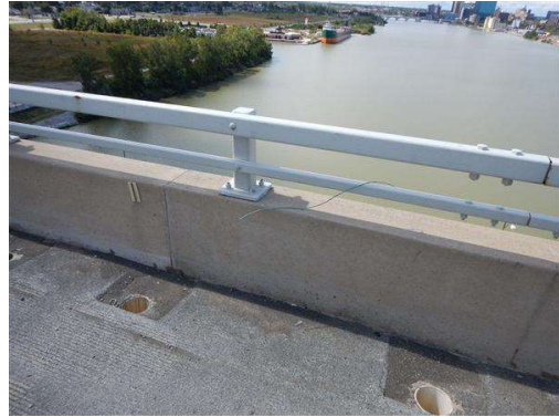
Photo 8 Disconnected grounding wire in Span 27SB
