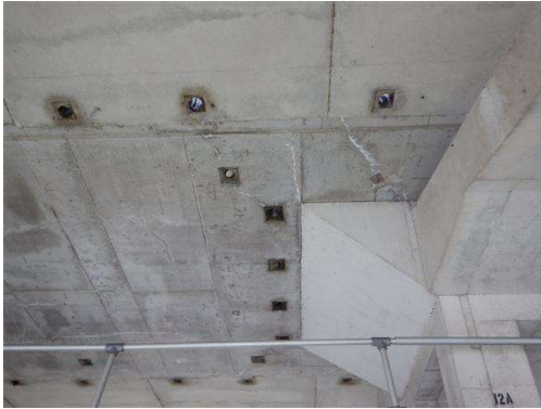
Photo 1 Transverse cracks with efflorescence in the bottom of the deck slab in Span 28NB
