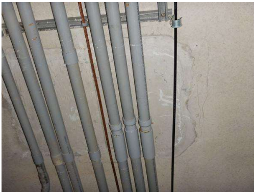
Photo 39 Construction access hole patch with cracks and efflorescence in Span 27SB
