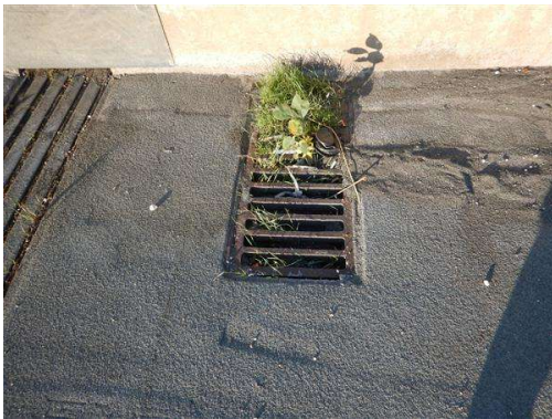
Photo 27 Scupper filled with debris and growing vegetation at Pier 29SB
