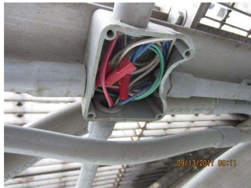
Photo 12 Missing cover on a damaged junction box exposing wires
