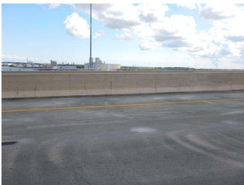
Photo 17 Typical hairline vertical cracks in the East parapet of Span 28SB looking East
