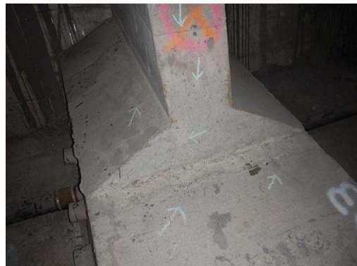
Photo 12 Multiple hairline cracks in deviator wall at Pier 27NB looking West
