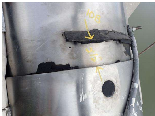
Photo 24 2.5" gap between sealant and top splice of Cable Stay 10B upper sleeve
