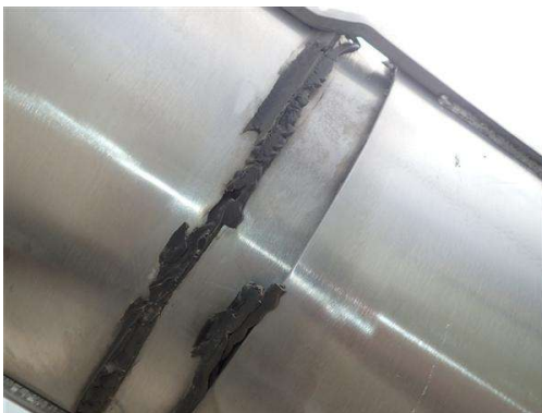
Photo 23 Full perimeter 2" gap in caulk at the top splice of Cable Stay 5B upper sleeve
