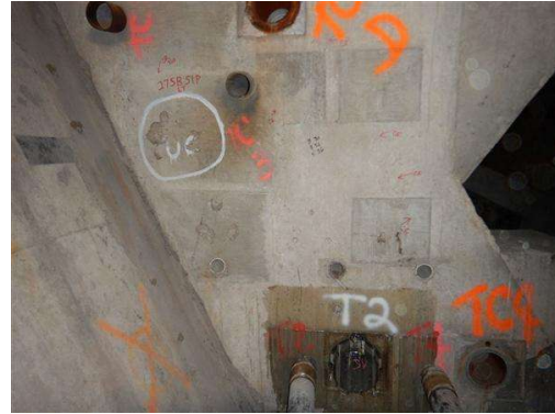
Photo 56 Cracks and spalls in the vertical face of the diaphragm at Pier 27SB
