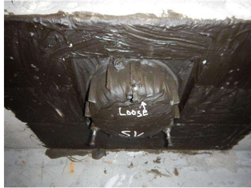
Photo 2 Loose bolt on PT anchor cap at Pier 28NB
