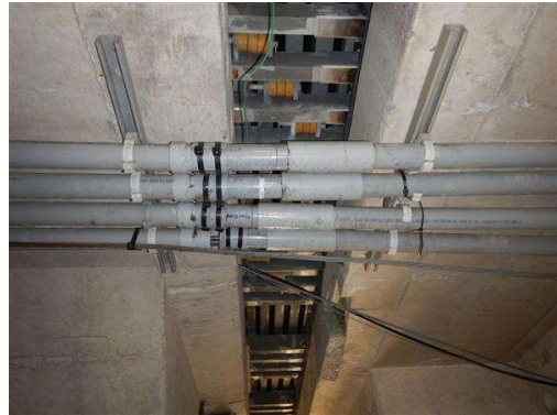
Photo 4 Separated electrical conduits and broken clamps at Pier 26NB
