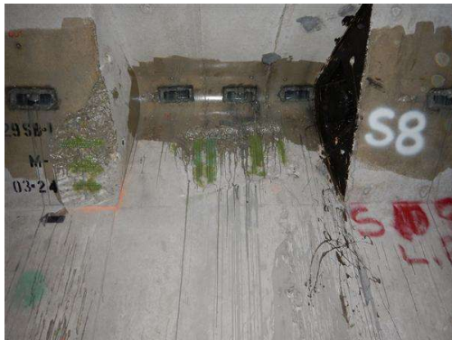
Photo 33 Typical spall with exposed reinforcement in the exterior PT block and web along the length of the bridge
