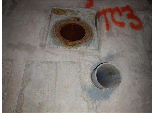
Photo 8 Typical rust on the future PT ducts on diaphragms looking Northeast
