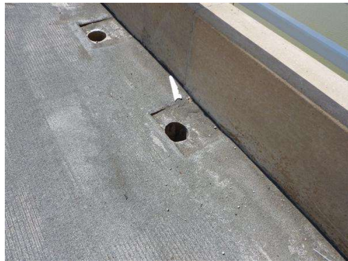
Photo 28 Missing PVC pipes in the drain holes on the West side of Span 27SB
