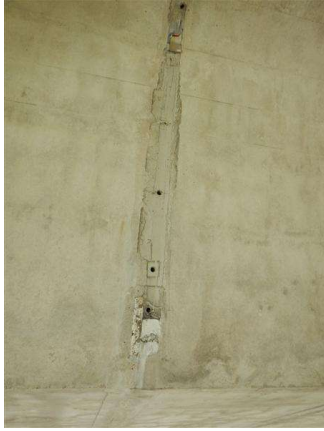
Photo 43 Multiple holes in closure pour between Segments 22 and 23 of Span 28SB
