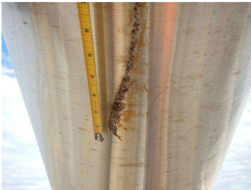
Photo 21 Gouge (8"x0.75") with light surface corrosion along the bottom side of the main sheath approximately 50' from the deck anchorage on Cable Stay 16A
