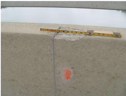
Photo 15 Spalls on the top of the East parapet in Span 27NB looking East
