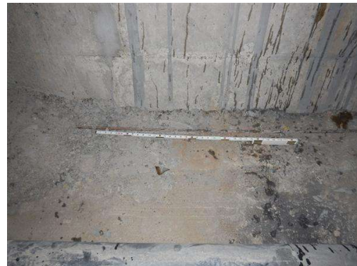
Photo 4 Exposed strand on the bottom flange/slab at Pier 27NB looking West
