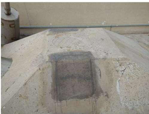
Photo 11 Delaminated/unsound concrete patch on the top face of deck Stay Cable Anchor 20A
