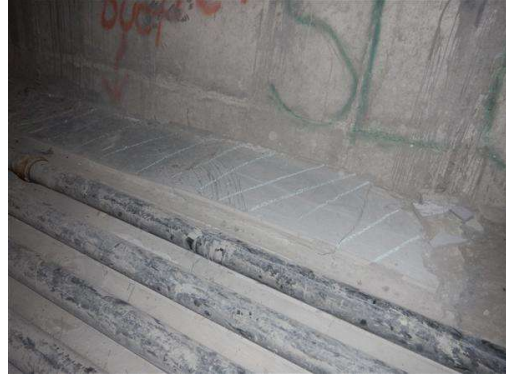
Photo 8 Delaminated concrete patch on the bottom flange/slab at Pier 27NB looking East
