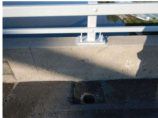
Photo 22 Spall in the West parapet in Span 28SB looking West
