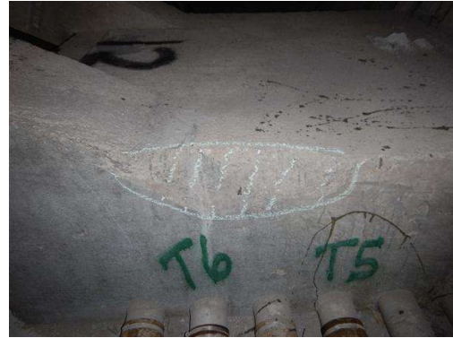
Photo 14 Spalls on the top edge of delta strut in Span 27NB
