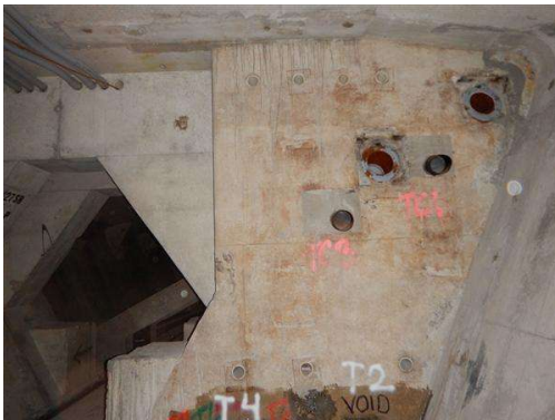
Photo 9 Typical rust on future PT ducts on the diaphragms
