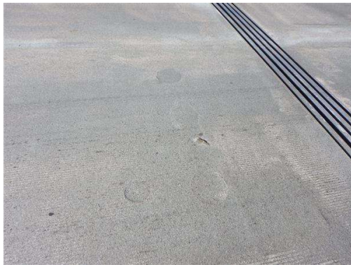
Photo 9 Concrete patches in the West traffic lane of Span 26SB
