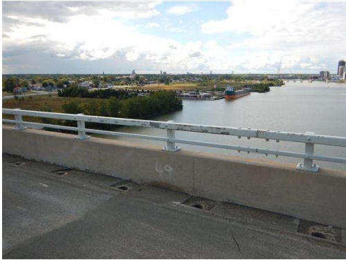
Photo 25 Coating damage/failure to the West steel railing in Span 27SB
