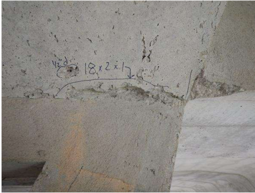
Photo 13 Spall (18"x2"x1") on South face (East side) of deck Stay Cable Anchor 18A
