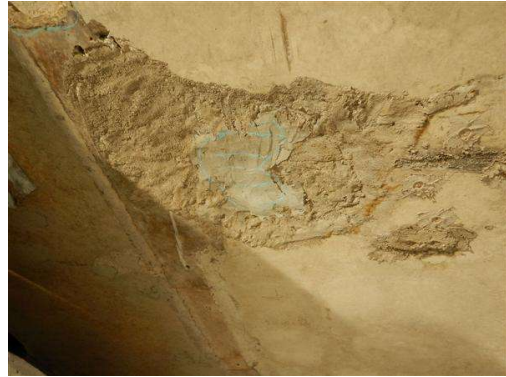
Photo 44 Delaminated concrete patch (14"x10") in the exterior bottom flange/slab of Span 26SB
