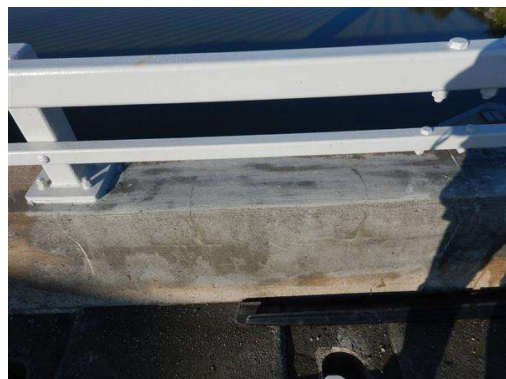
Photo 18 Cracks in the West parapet in Span 28SB looking West
