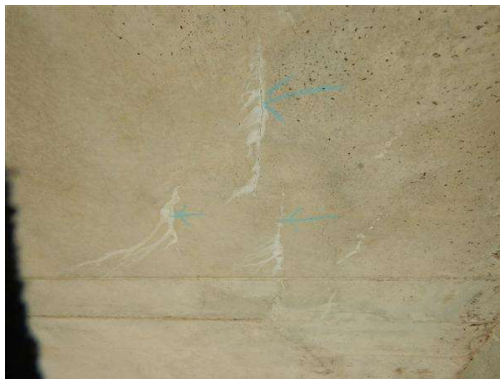
Photo 47 Longitudinal cracks with efflorescence in the exterior bottom flange of Span 28SB
