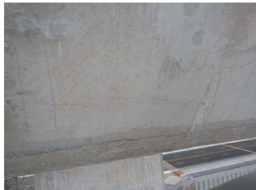
Photo 24 Typical longitudinal cracks on the exterior webs
