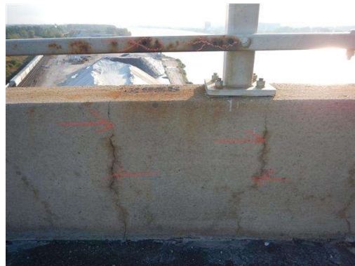
Photo 12 Full height vertical cracks in the East parapet in Span 28NB looking East
