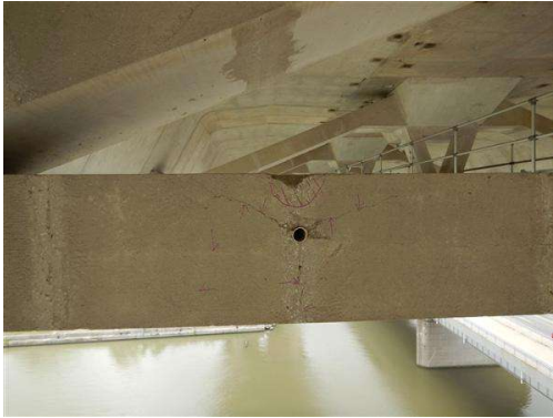
Photo 19 Spall and cracks in the lower right strut at Cable Stay Anchor 3B in Span 27NB
