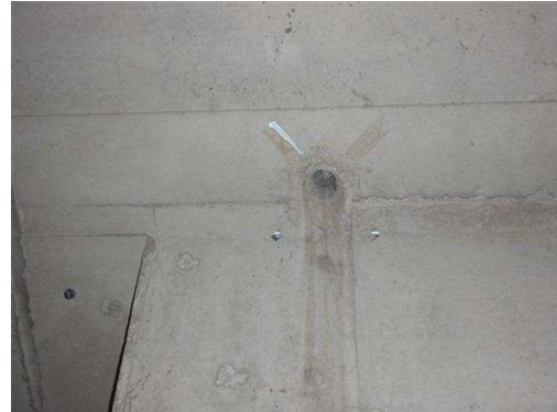
Photo 2 Lift hole missing grout in Span 28NB
