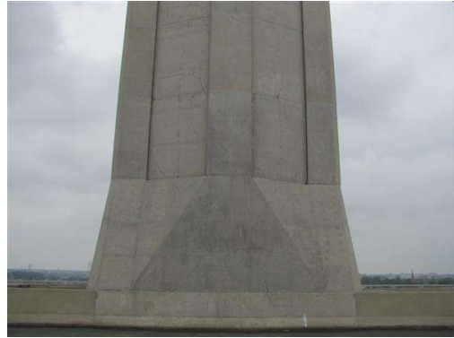
Photo 14 Leaching efflorescence on the West parapet in Span 28NB looking West
