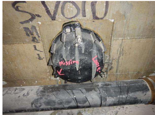
Photo 4 Loose and missing bolt on PT anchor cap in Span 27SB
