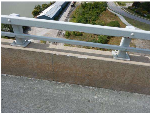
Photo 23 Gouges and 2" saw cut unfilled in Span 29SB of West parapet
