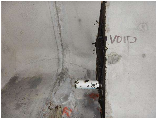
Photo 21 Typical interior, upper corner cracks along the length of the bridge looking East
