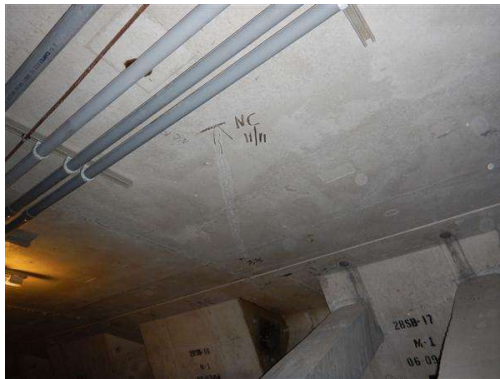
Photo 45 Longitudinal cracks with efflorescence in the top flange/slab of Span 28SB
