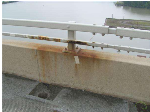
Photo 16 Deterioration and heavy rust in the East steel railing of Span 27NB looking East
