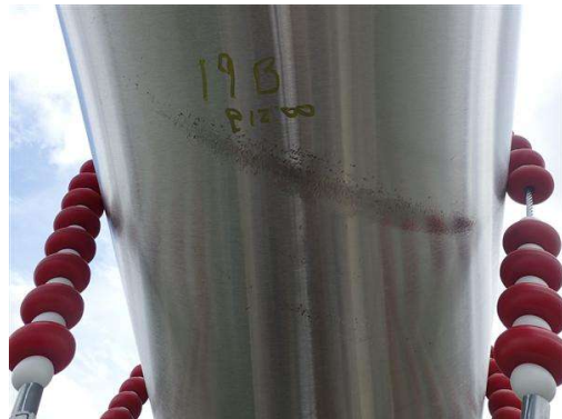
Photo 22 Scrape/surface gouge (12"x3") along the bottom face of the main sheath, near the upper splice on Cable Stay 19B
