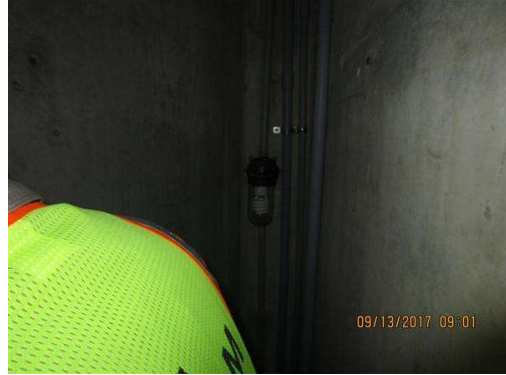
Photo 14 Burned out service lights in the personnel liftway
