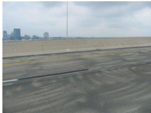
Photo 10 Scaling and abrasion in the wearing surface in Span 26NB looking West
