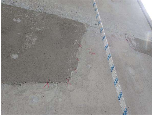
Photo 29 Two (2) patches with 0.0625" wide gaps along the bottom edge on the Upper Pylon West face near Cable Stay 20
