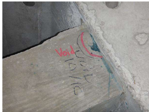
Photo 48 Small void at the intersection of strut and corner block in Span 28SB
