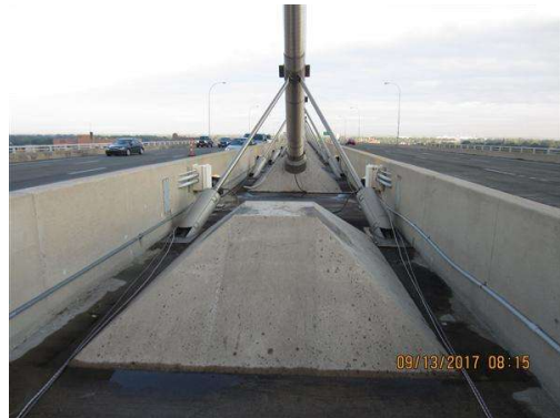
Photo 10 Typical hairline cracks on top of deck Stay Cable Anchors
