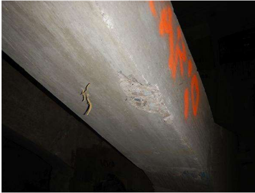
Photo 37 Typical spall in the strut legs along the length of the bridge
