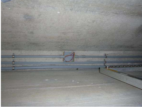
Photo 13 Missing junction box cover in the liftway
