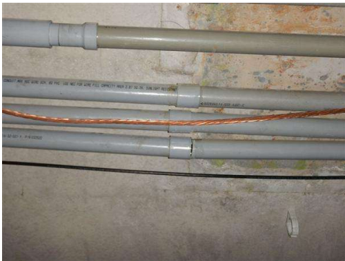
Photo 9 Separated electrical conduit in Span 27SB
