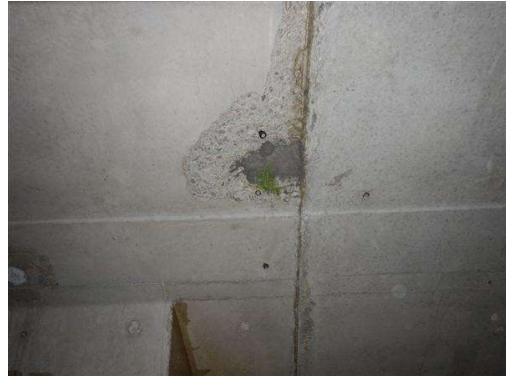
Photo 32 Spall with exposed reinforcement in the top flange/slab of Span 28SB
