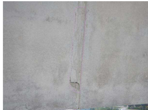
Photo 16 Spall (5"x7"x1") in the exterior East web of Span 28NB looking West
