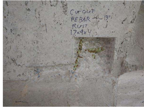
Photo 14 Concrete cutout with exposed reinforcement on the bottom (South face) of deck Stay Cable Anchor 16A
