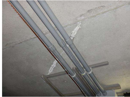
Photo 20 Cracks with leaching efflorescence in the top flange/slab in Span 28NB
