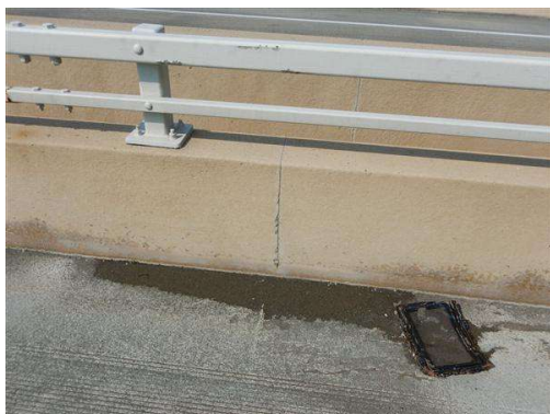
Photo 19 Typical minor paint damage on steel railing along the length of the bridge
