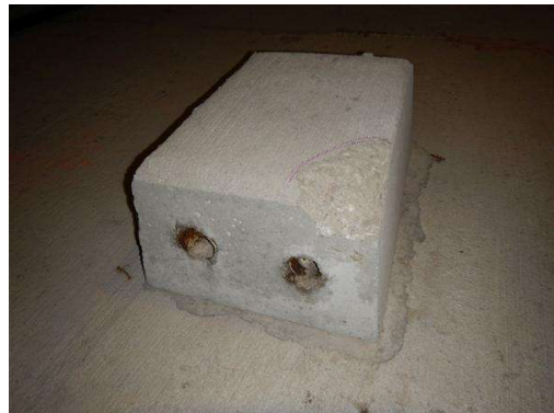
Photo 22 Spall on exterior floor PT stressing block in Span 34SB looking South
