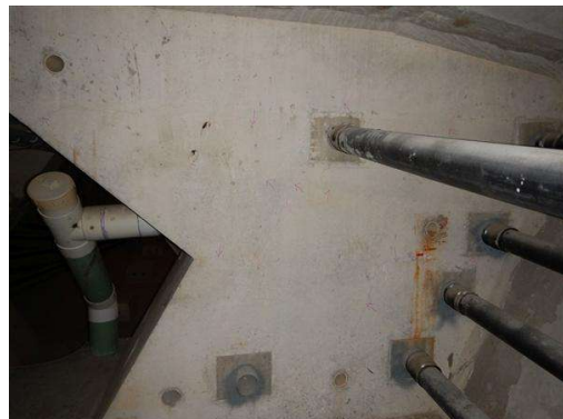
Photo 24 Map cracking and rust stains on vertical face of diaphragm at Pier 30SB looking South
