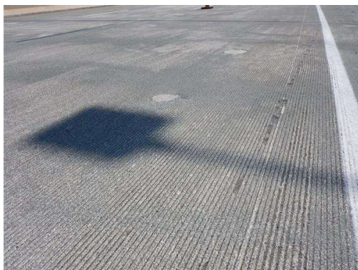
Photo 7 Scaling and damage to grooving (10') in Span 39SB
