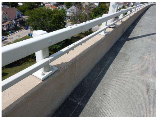
Photo 15 Minor spalls on the edge of the parapet in Span 37SB
