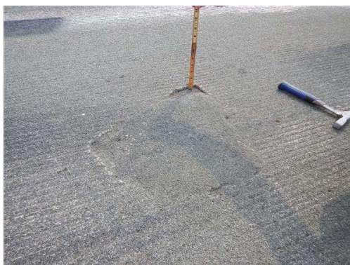
Photo 4 Spall (12"x12"x1") in Span 51SB
