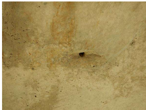
Photo 8 Spall at the drain hole in Span 36SB
