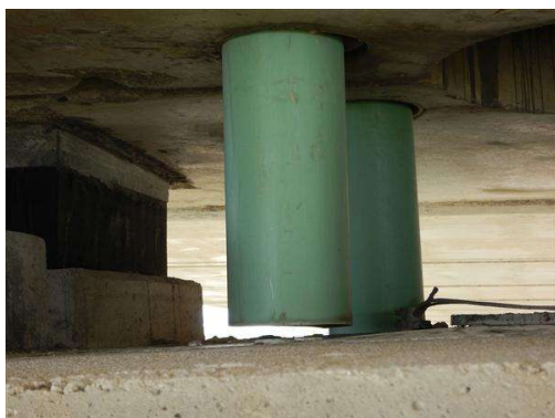
Photo 3 Drainage pipe on Southeast side at Pier 38SB does not extend into the cap
