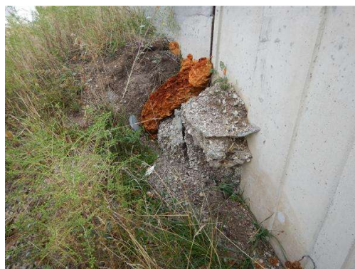
Photo 4 Erosion along wingwall at the back side of the approach slab
