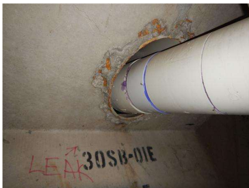
Photo 23 Interior drainage leak and minor rust stains at Pier 30SB
