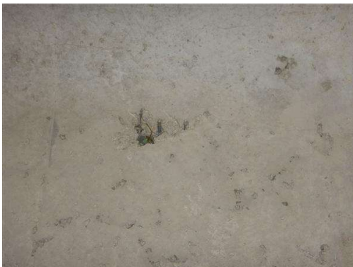
Photo 23 Typical honeycombed concrete in the webs looking East
