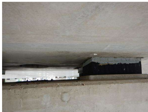
Photo 28 Vertical cracks in the plinth of East bearing at Pier 51SB
