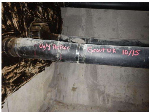
Photo 5 Poor sheathing work on PT duct in Span 39SB looking West
