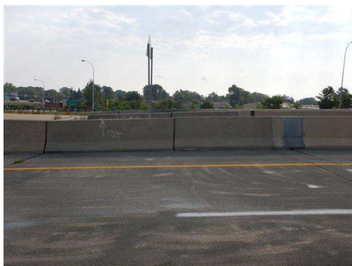
Photo 5 East barrier displaced/rotated by 0.75" looking East
