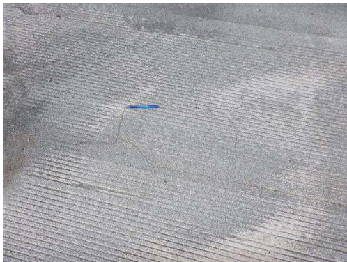
Photo 2 Map cracking along closure pour in Span 48SB
