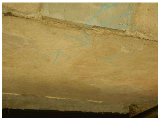
Photo 15 Cracks in the bottom flange at Pier 38SB
