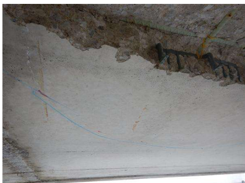
Photo 9 Spall of (5'x20.5'x3.5') in the bottom flange of Span 52SB
