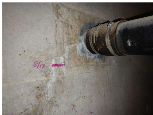
Photo 4 Leaching efflorescence from PT duct in Span 44SB
