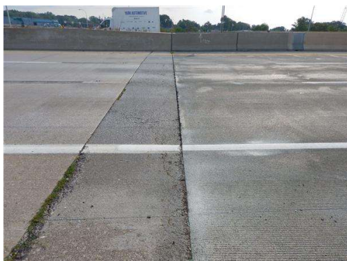
Photo 3 Cracks and growing vegetation in relief joint looking East
