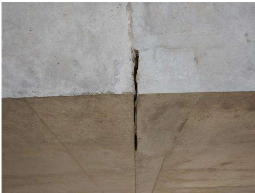
Photo 21 Missing epoxy/joint filler between Segments 12 and 13 in Span 37SB
