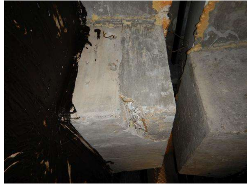
Photo 2 Spall with exposed reinforcement in the PT block in Span 48SB
