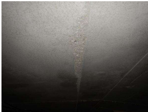
Photo 3 Typical spall in the top flange/slab in Span 30SB
