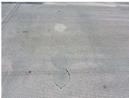
Photo 6 Liftholes with spalls around perimeter in Span 48SB
