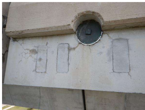
Photo 12 Concrete patches with cracks, efflorescence and discoloration on PT end block at Pier 36SB
