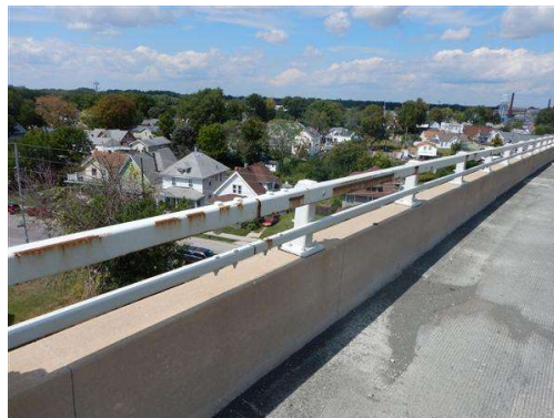
Photo 18 Typical condition of the steel railing with rust staining and minor deterioration along the length of the bridge
