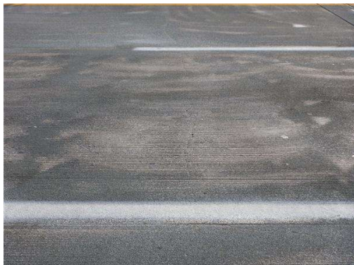
Photo 1 Transverse crack in the traffic lane of approach slab looking East
