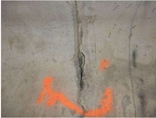
Photo 19 12" deep void in the interior segment joint in Span 34SB
