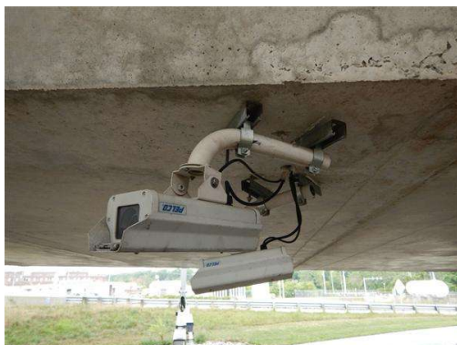
Photo 5 Loose security camera bracket in Span 58SB
