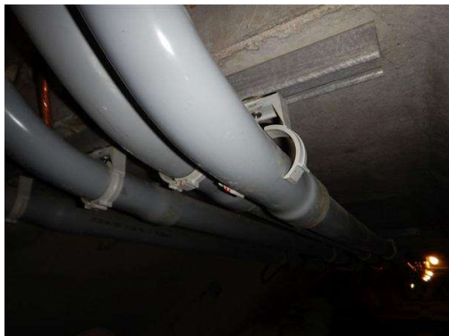
Photo 1 Broken electrical conduit bracket in Span 33SB
