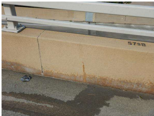
Photo 17 Typical spalls in the vertical joint of the West parapet looking West
