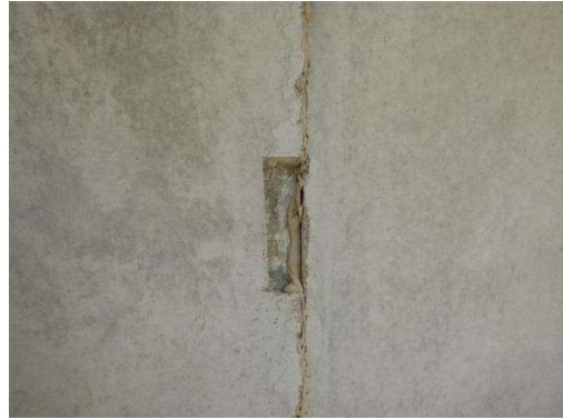
Photo 20 Concrete cut out (9"x3"x1.5") in the web in Span 34SB
