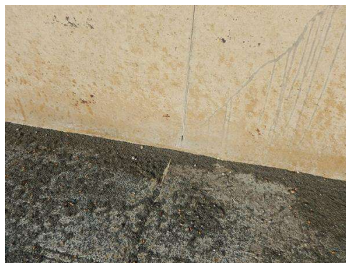
Photo 12 Bottom of saw cut in the West parapet in the Span 33SB was not filled
