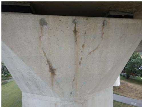
Photo 2 Typical vertical and longitudinal cracks with rust stains in the pier caps
