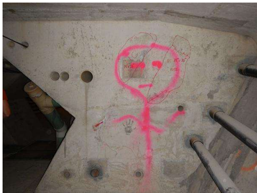
Photo 25 Delaminated concrete in the vertical face of the diaphragm at Pier 47SB looking North
