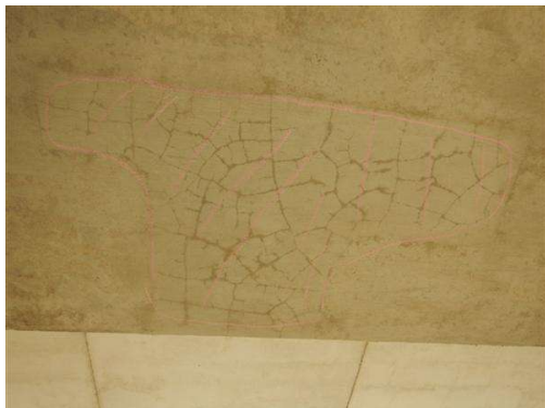
Photo 7 Delaminated patch with discoloration in the web in Span 57SB
