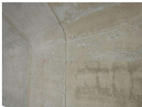
Photo 16 Typical longitudinal and map cracks with efflorescence in the exterior webs
