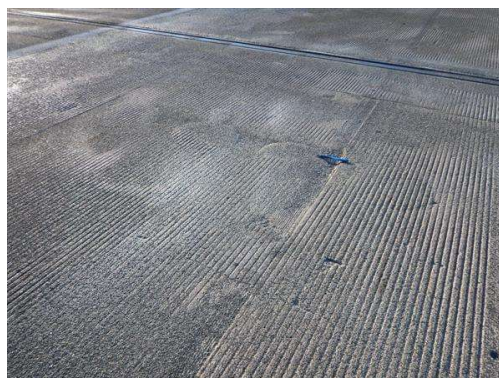
Photo 10 Depression (0.375\") in deck/wearing surface in Span 35SB
