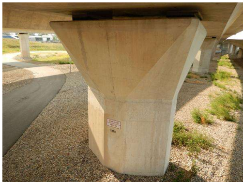
Photo 1 Typical honeycombed and hairline cracks on the columns
