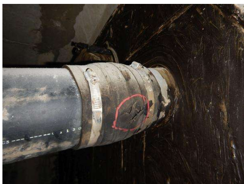
Photo 3 Tear in the PT duct splice at Pier 36SB looking West
