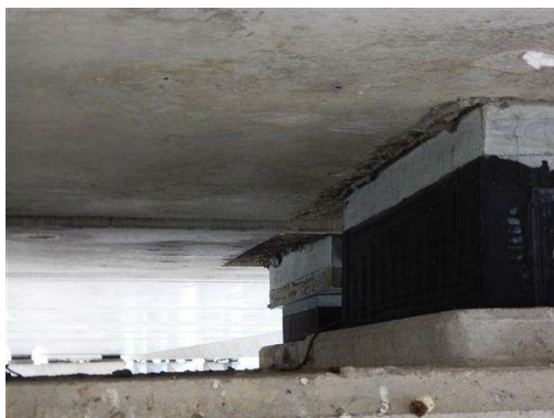
Photo 29 Honeycombed concrete around the edges of each bearing at Pier 51SB
