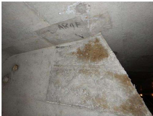
Photo 5 Crack in the top of the deviator wall in Span 32SB
