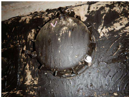
Photo 1 Voids in the PT anchor cap at Pier 39SB looking South
