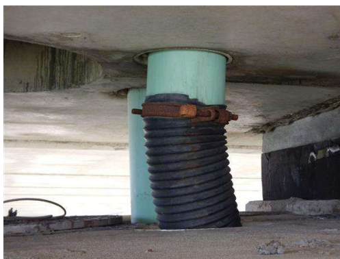
Photo 4 Heavy rust on drainage pipe clamp at Pier 38SB
