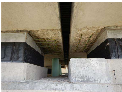
Photo 11 Spall of (3.5'x12'x2') in the bottom flange at bearings at Pier 36SB
