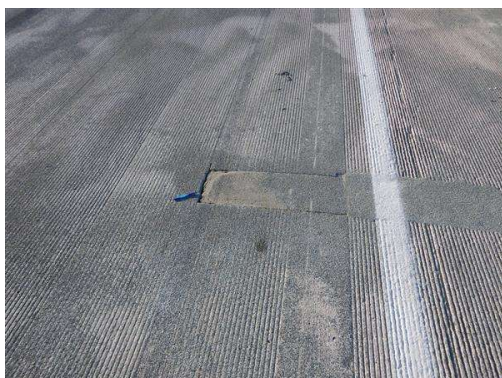
Photo 3 Concrete patch with 0.5" deep spall in Span 35SB
