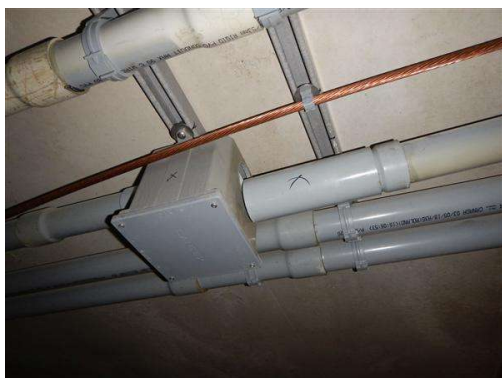
Photo 3 Loose electrical conduit in Span 48SB
