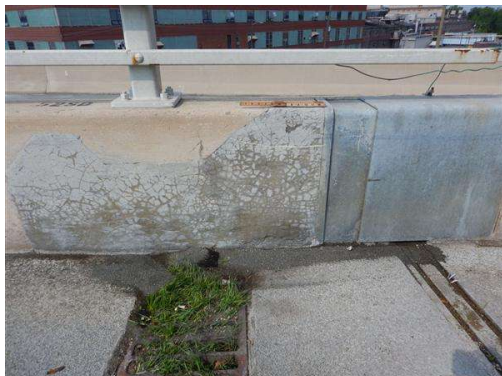
Photo 13 Delamination and vertical cracks on face of the West parapet in Span 51SB looking West
