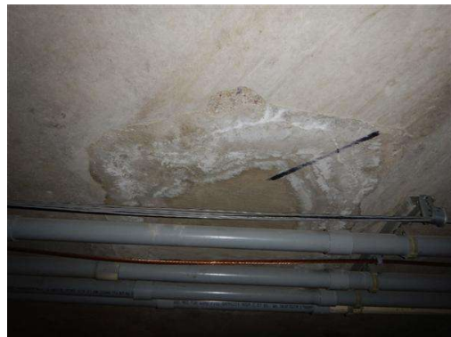
Photo 6 Construction access hole patch with spalls and efflorescence in Span 37SB
