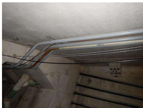
Photo 4 Loose/hanging cables in Span 56SB looking West
