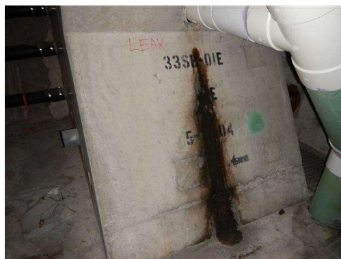
Photo 22 Interior drainage pipe at Pier 33SB with rust staining
