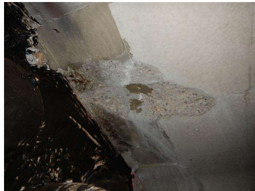
Photo 4 Spall in the top flange/slab in Span 41SB
