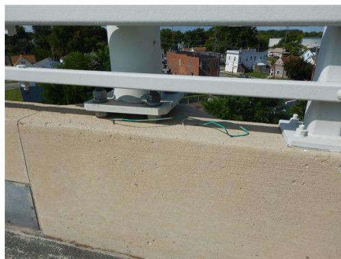
Photo 6 Disconnected grounding wire in Span 44SB
