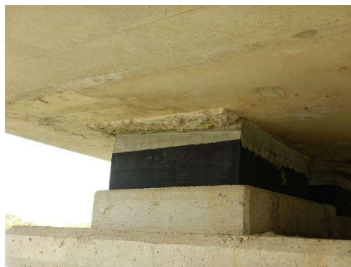
Photo 30 Spalls with exposed reinforcement at North bearing at Pier 38SB
