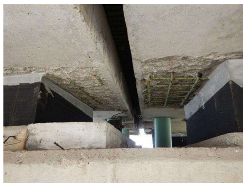
Photo 10 Spall with exposed reinforcement in the bottom flange at Pier 33SB bearings
