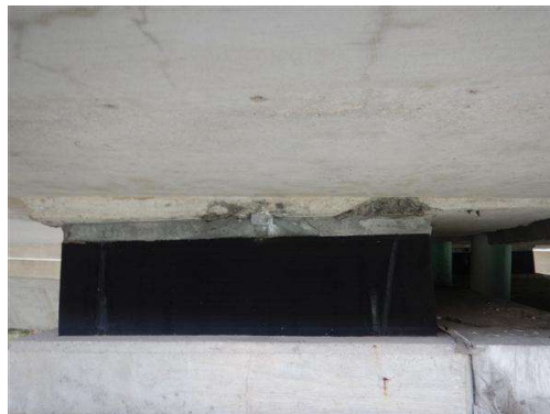
Photo 26 Spall in the West bearing plinth at Pier 56SB
