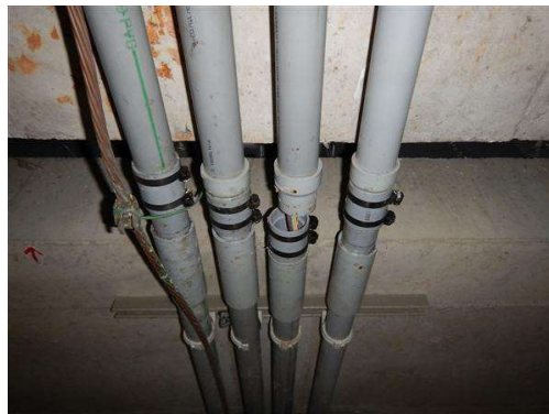
Photo 2 Separated electrical conduits in Span 30SB looking South
