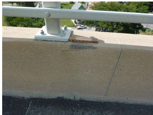
Photo 14 Delamination in parapet beneath the steel railing post in Span 37SB looking West
