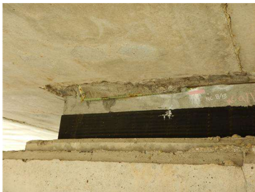
Photo 27 Spalls with exposed reinforcement at East bearing at Pier 34SB
