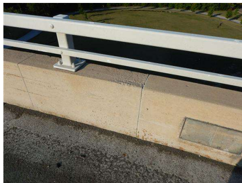
Photo 16 Scaling on the top of the West parapet in Span 34SB
