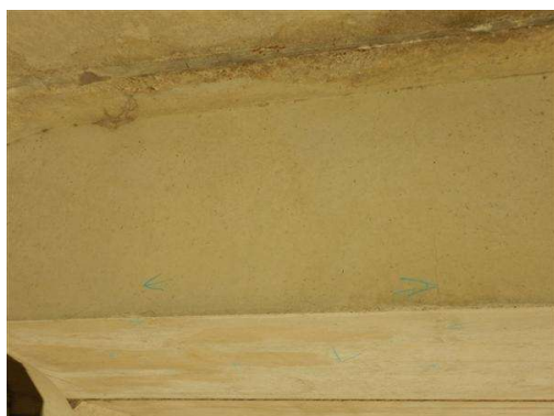
Photo 17 Full height vertical cracks on South face of PT pier end segment at 38SB
