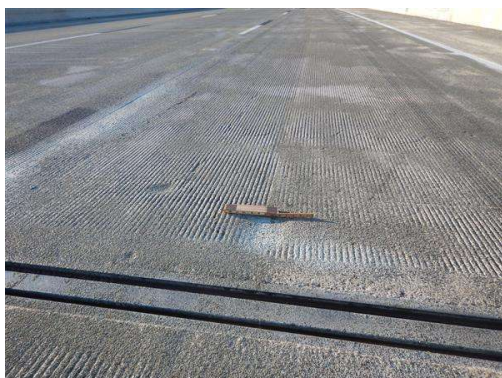
Photo 9 Depression (0.25\") in deck/wearing surface in Span 36SB
