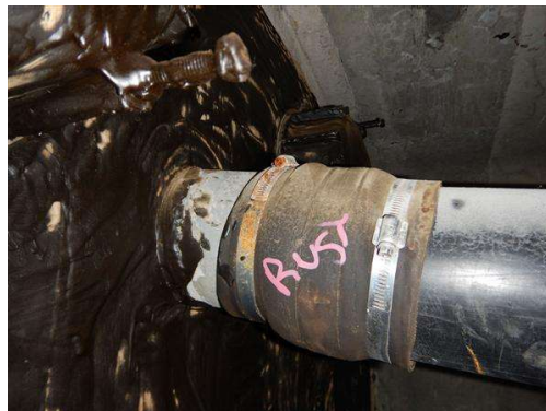
Photo 2 Rust on PT duct clamp at Pier 51SB looking West
