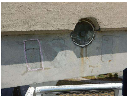
Photo 21 Rust stains and efflorescence on the edge face of the end segments along with delaminated concrete patches
