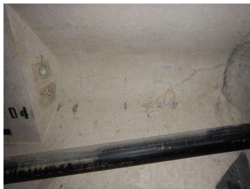
Photo 14 Interior upper corner cracks typical along the length of the bridge
