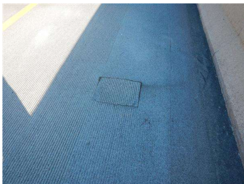
Photo 5 Concrete patch with spalls and discoloration around perimeter in the shoulder in Span 31SB
