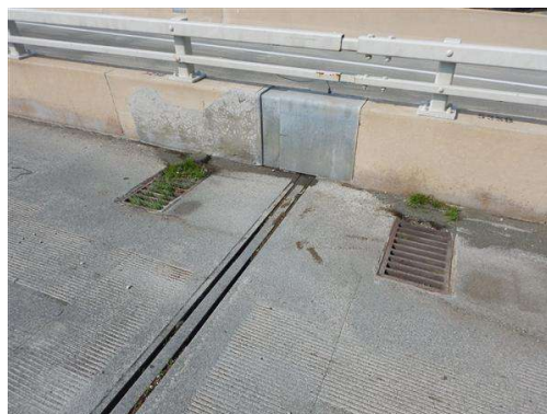
Photo 20 Fully filled scuppers with vegetation growing in Span 52SB looking West
