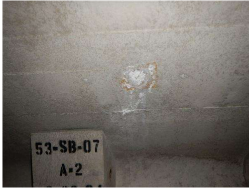
Photo 1 Efflorescence leaching from lift holes in Span 53SB
