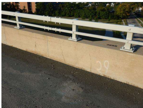
Photo 11 Typical full height vertical cracks in the West parapet looking West
