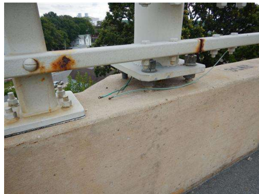
Photo 6 Disconnected grounding wire in Span 39NB
