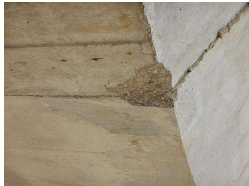
Photo 10 Spall (8"x8"x0.5") between Segments 12 & 13 in Span 34NB
