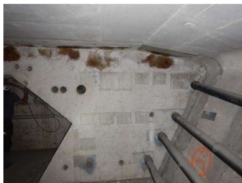
Photo 22 Map cracking and rust stains on vertical face of diaphragm at Pier 58NB
