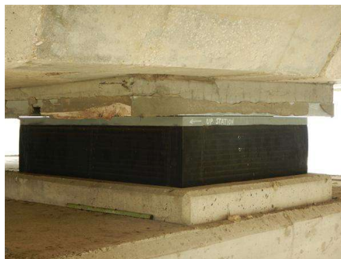
Photo 24 Gap between load plate and sole plate on West bearing at Pier 29NB looking South
