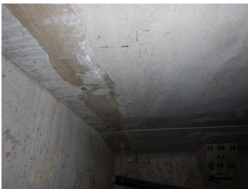
Photo 11 Cracks with efflorescence in the top flange in Span 35NB
