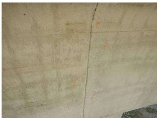
Photo 15 Typical hairline longitudinal cracks in the exterior webs
