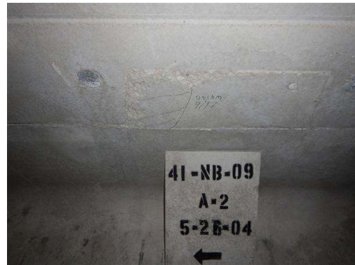
Photo 4 Delamination in the top flange over future PT block in Span 41NB
