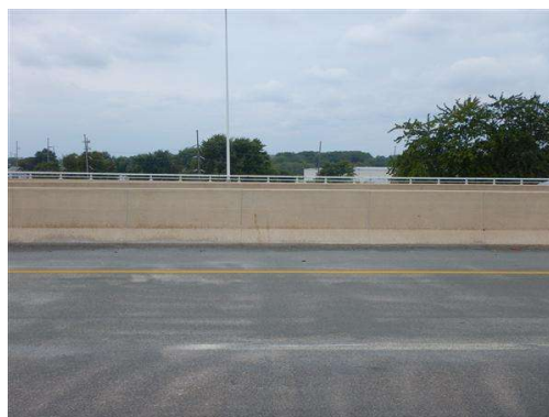
Photo 10 Typical vertical cracks in the West parapet looking West
