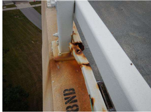
Photo 20 Deterioration in the steel railing due to heavy rust in Span 38NB
