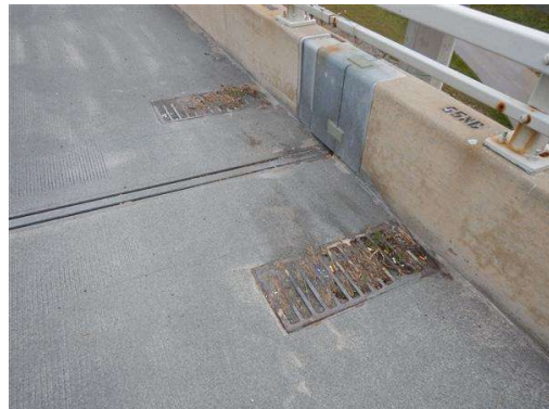
Photo 22 Fully filled scuppers with vegetation growing at Pier 55NB looking East
