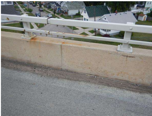
Photo 15 Delamination in East parapet in Span 43 looking East
