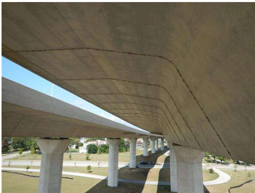
Photo 9 Grout or epoxy leakage between segments in Span 34NB looking North
