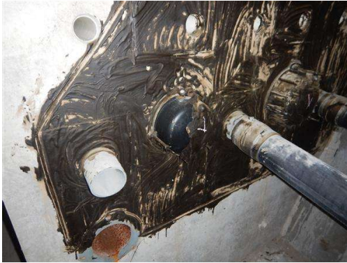
Photo 1 Voids in the PT anchor cap
