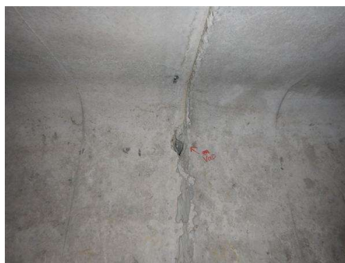
Photo 18 9" deep void in the interior construction joint in Span 44NB
