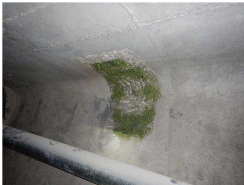
Photo 5 PT block removed with exposed reinforcement in Span 43NB
