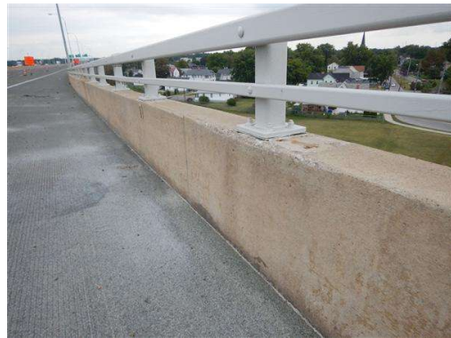
Photo 16 Scaling along the top of East parapet in Span 40NB looking East
