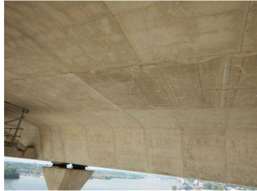
Photo 2 Bottom of the deck slab closure pour with transverse cracks and efflorescence in Span 29NB
