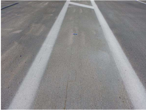
Photo 1 Hairline to moderate (0.025") cracking with efflorescent leaching in closure pour joint
