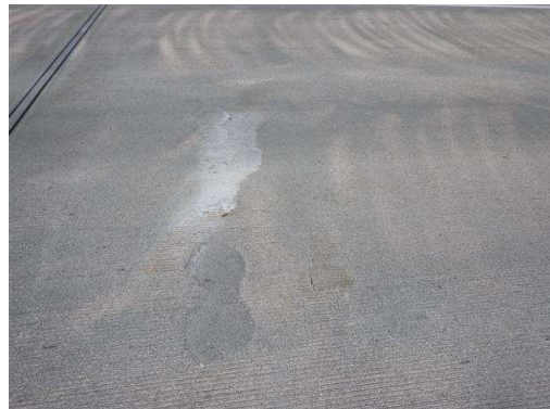
Photo 4 Lift hole patches with spalling and efflorescence around the perimeter at Pier 56NB
