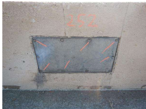
Photo 4 Missing and loose screws in the electrical panel in Span 31NB
