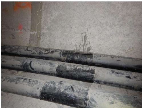
Photo 5 Splice material not properly adhered to the PT tendon in Span 55NB
