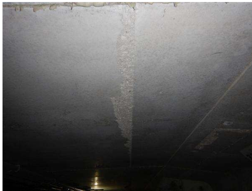
Photo 3 Concrete spall (5"x6"x1") in the top flange/slab in Span 33NB
