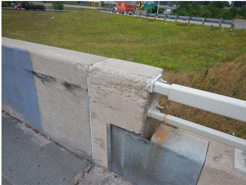
Photo 3 Concrete spall 21"x8"x3/4" in East parapet looking East
