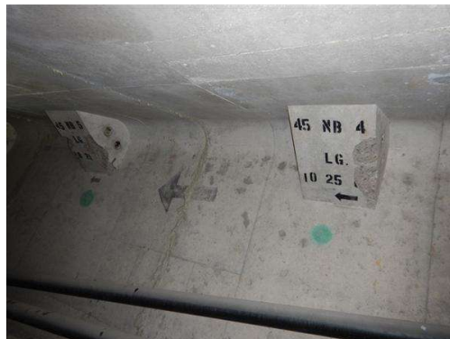
Photo 20 Typical concrete spalls in the future PT blocks
