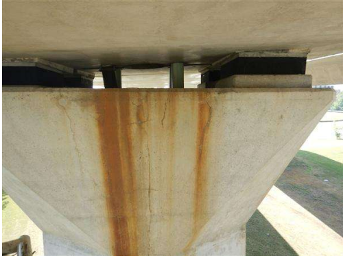
Photo 1 Typical cracking and efflorescence or staining in the pier caps
