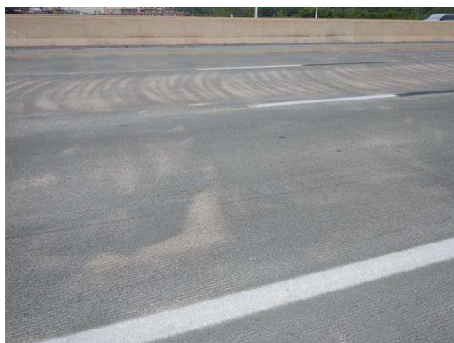
Photo 9 Scaling and abrasion in the wearing surface looking West
