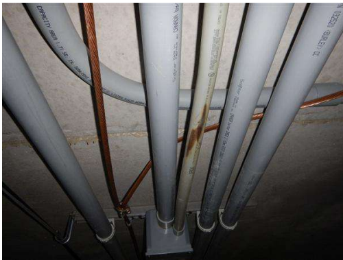
Photo 3 Burned electrical conduit in Span 54NB
