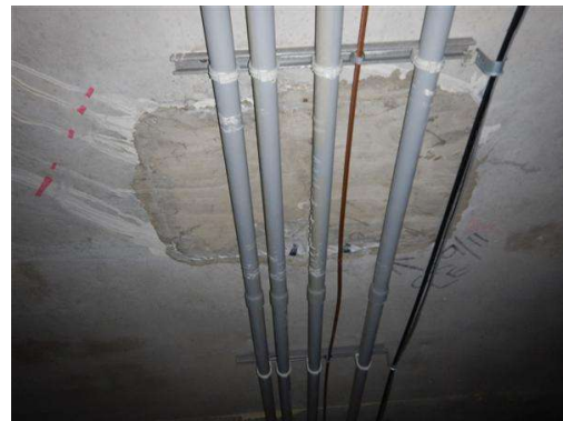
Photo 6 Construction access hole patch cracks and efflorescence in Span 33NB
