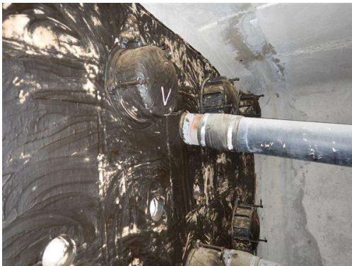
Photo 3 Rust on PT duct at Pier 52NB
