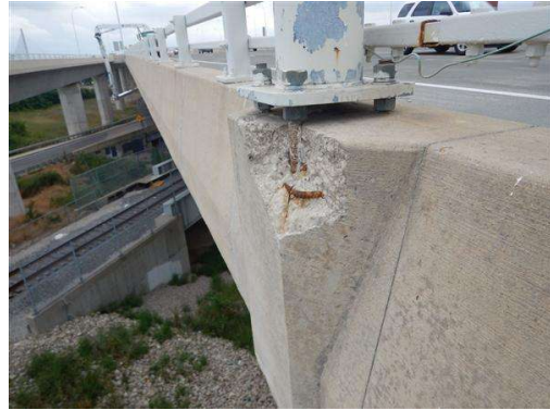
Photo 14 Spall at the light pole with exposed reinforcement in Span 55NB looking South
