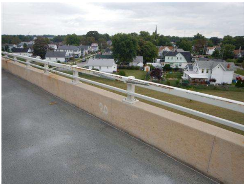
Photo 21 Paint damage to the steel railing in Span 41NB looking East
