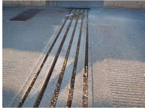
Photo 26 Pier 30NB expansion joint fully filled with debris looking East
