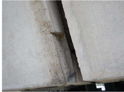
Photo 8 Concrete cut out of the web at the end of the beam at Pier 45NB looking West
