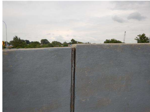
Photo 4 0.75" header gap between concrete barriers looking East
