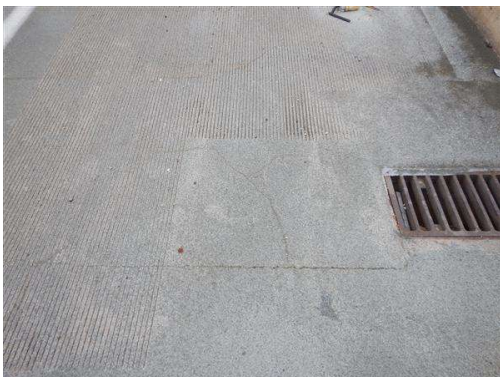
Photo 5 Unsound concrete patch (1'x1') with map cracking at Pier 45NB scupper
