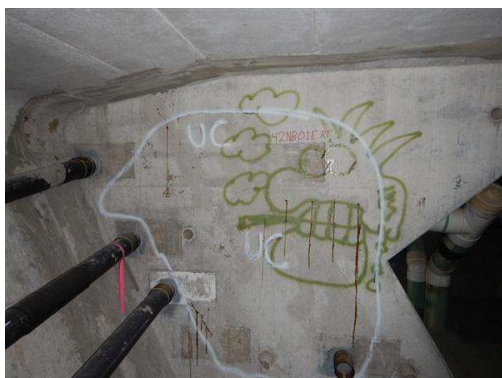
Photo 21 Delaminated concrete area in the vertical of the diaphragm at Pier 42NB
