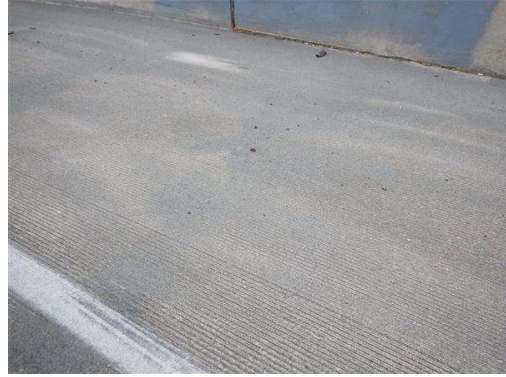
Photo 2 Transverse cracks in East side of the approach slab looking East
