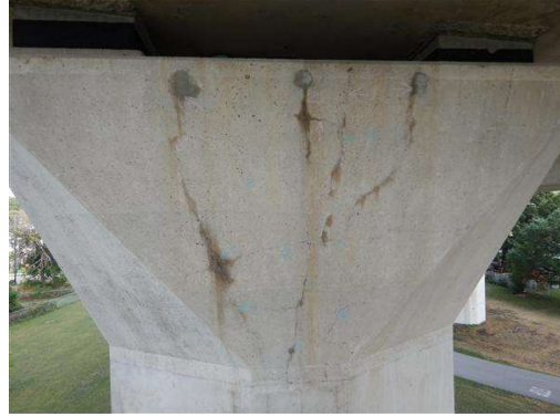
Photo 2 Typical cracking and efflorescence or staining in the pier caps
