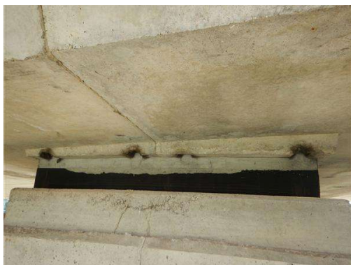
Photo 23 Concrete spalls in East bearing plinth of Pier 37NB
