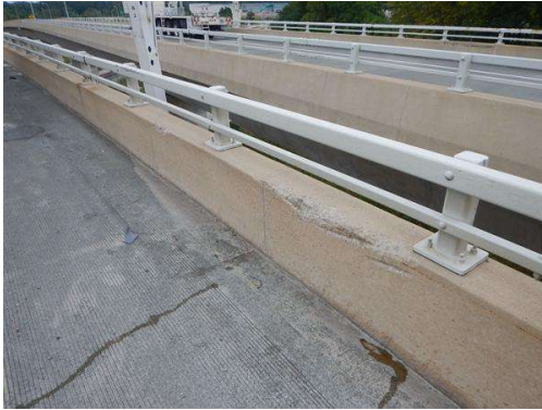
Photo 13 Spall (42"x15"x2") on the East parapet in Span 53NB looking East
