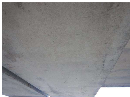
Photo 16 Longitudinal and transverse cracks in the bottom of PT block at Pier 42NB
