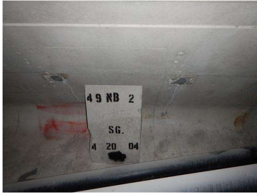
Photo 1 Efflorescence leaching from lift holes in Span 49NB
