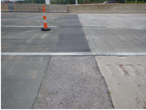
Photo 1 Concrete spalls in approach pavement in all lanes looking West
