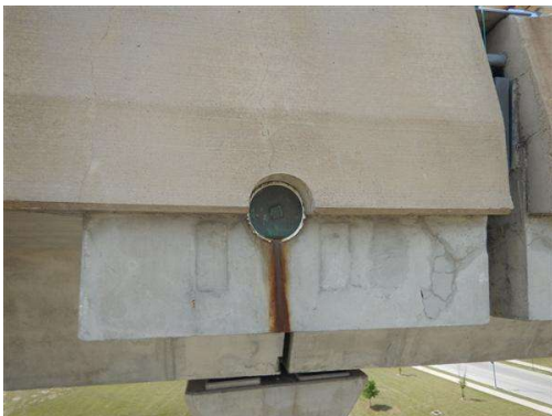
Photo 23 Heavy rust staining and efflorescence on the edge face of the end segments
