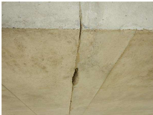
Photo 19 Void in the exterior construction joint in the bottom flange in Span 39NB
