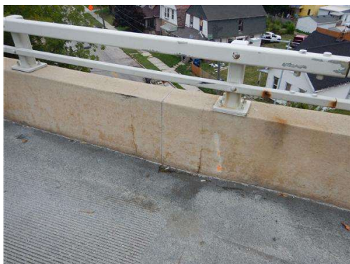
Photo 11 Typical full length vertical cracks in the East parapet looking East
