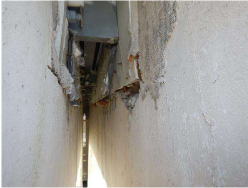
Photo 7 Spall (8"x3"x1.5") in PT block 2 at Pier 42NB looking West
