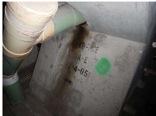
Photo 24 Interior drainage pipe at Pier 32NB with rust staining
