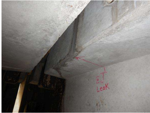
Photo 25 Leaking expansion joint at Pier 53NB
