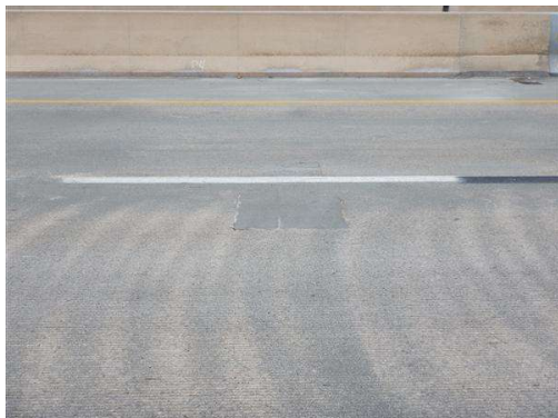
Photo 7 Delaminated concrete patch (5'x3') in the West traffic lane in the Span 55NB looking West
