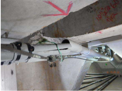
Photo 1 Broken and separated electrical conduit in Span 30NB
