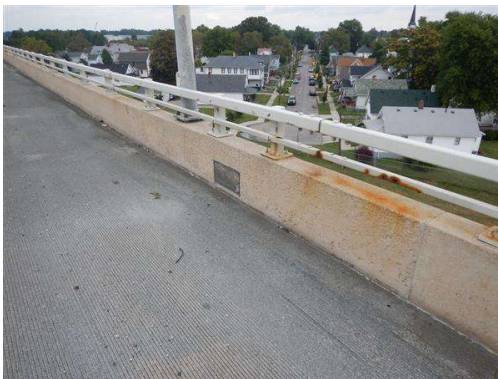
Photo 17 Concrete popouts in East parapet in Span 42NB looking East
