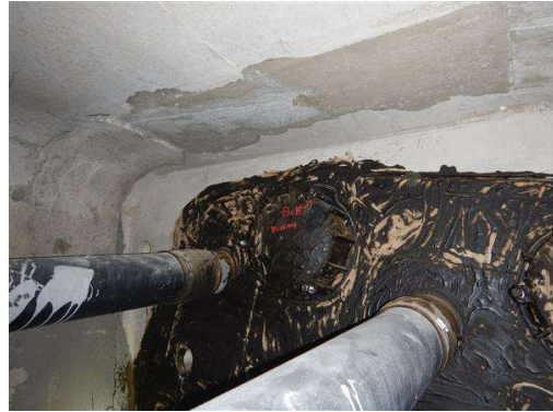
Photo 2 Missing bolt on PT anchor heads and rust on clamps at Pier 55NB
