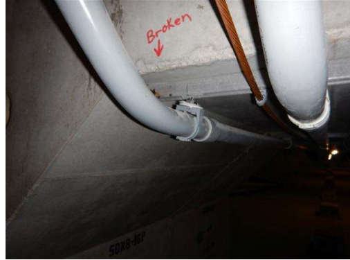
Photo 2 Broken electrical conduit bracket in Span 50NB
