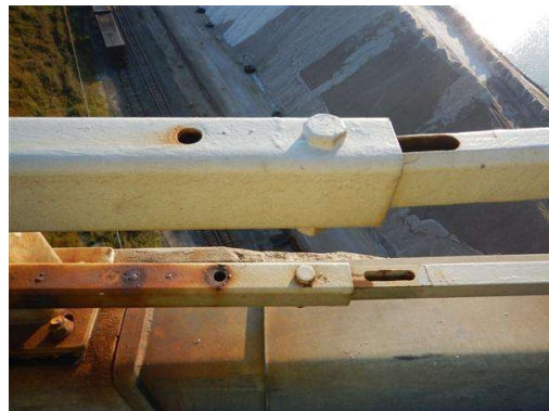
Photo 18 Missing splice plate bolt for the steel railing in Span 30NB looking East
