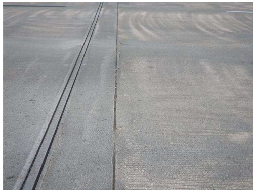
Photo 27 Concrete spalls in the expansion joint header at Abutment 59NB looking West
