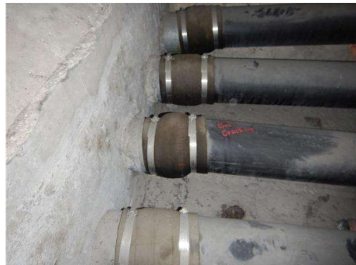
Photo 4 Cracking and bulging on PT sleeves at Pier 58NB
