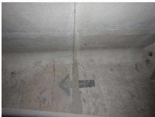
Photo 13 Interior upper corner cracks typical along the length of the bridge
