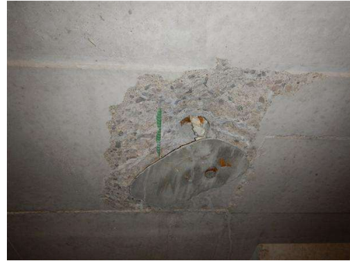
Photo 2 Severe spall at lift hole location with exposed reinforcement in Span 50NB
