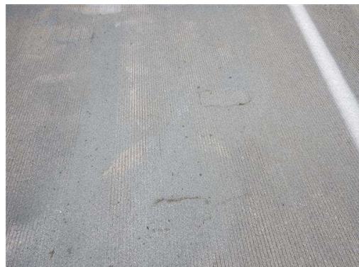
Photo 6 Concrete patches with minor spalls around the perimeter in the Span 45NB
