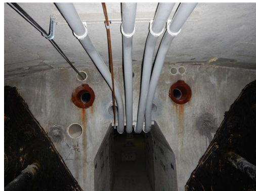
Photo 6 Typical rust on the future PT ducts located in the diaphragms
