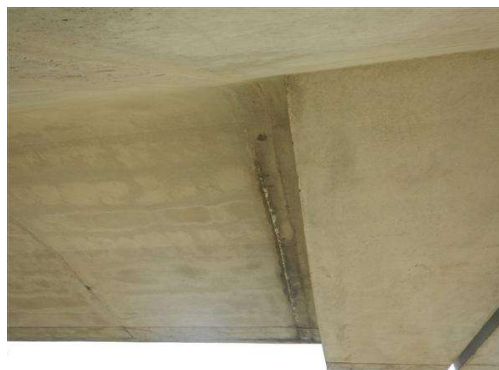
Photo 14 Cracks with efflorescence in the cantilever portion of the slab at Pier 36NB looking East
