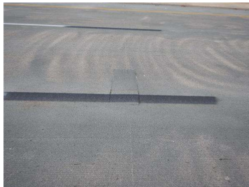
Photo 8 Concrete patch with map cracking in the travel lane in Span 58NB looking West
