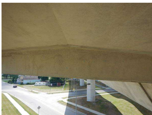
Photo 17 Typical cracking in the vertical faces of the PT end segments at the piers
