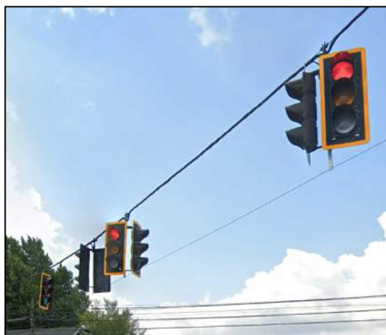
Photo 3: Intersection Span Wire
