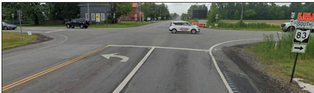
Photo 2: Signage and Pavement Marking Conditions, SR 83 Looking South
