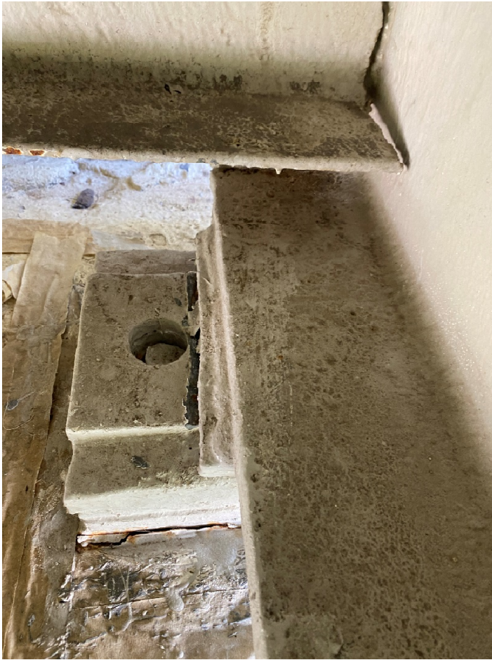
Photo # 19: Lateral displacement of beam 5 bearing at forward abutment. This bearing is furthest from the collision point.
