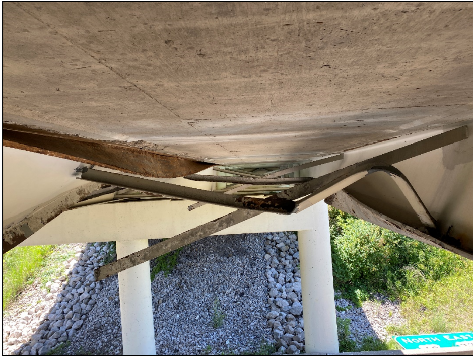
Photo # 7: Bay 1 crossframe 3 (fore) damage looking south.
