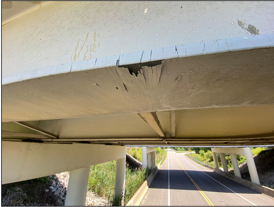
Photo # 13: Stress cracks in paint from lateral deflection at crossframe 4, span 2, beam 1
