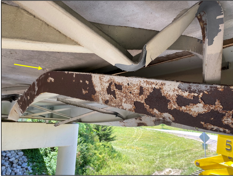
Photo # 9: Beam 2 distortion at point of impact – note damage to deck from beam bottom flange.
