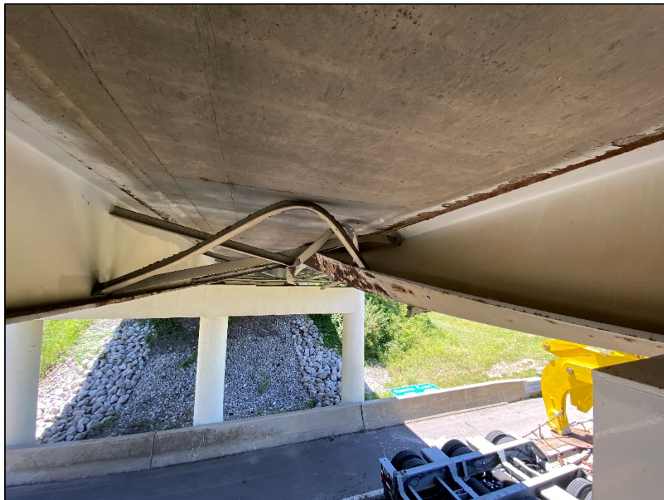
Photo # 12: Bay 2, crossframe 3 damage.
