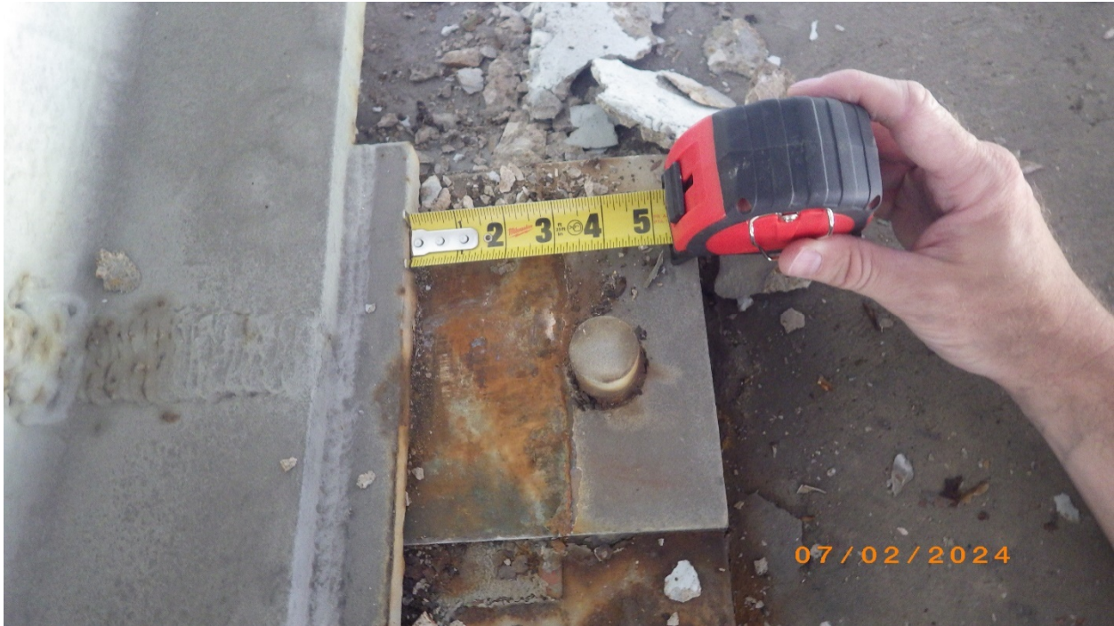
Photo # 17: Lateral displacement from collision, beam 2 bearing over pier 1.
