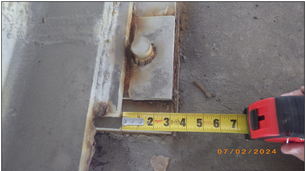
Photo # 16: Lateral displacement of beam 3 bearing over pier 1.
