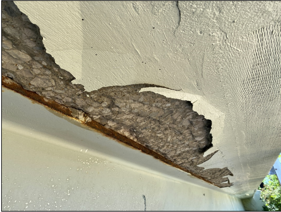
Photo # 5: Beam 1 top flange gap with spalled deck cantilever.
