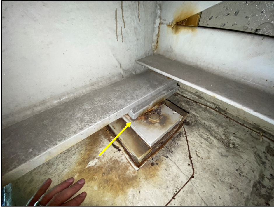
Photo # 15: Displacement of bearing 4 at rear abutment. (Typical to interior beams at rear abutment.)
