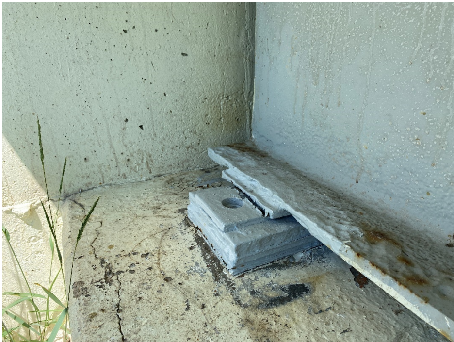
Photo # 18: Lateral displacement from collision, beam 2 bearing at forward abutment.
