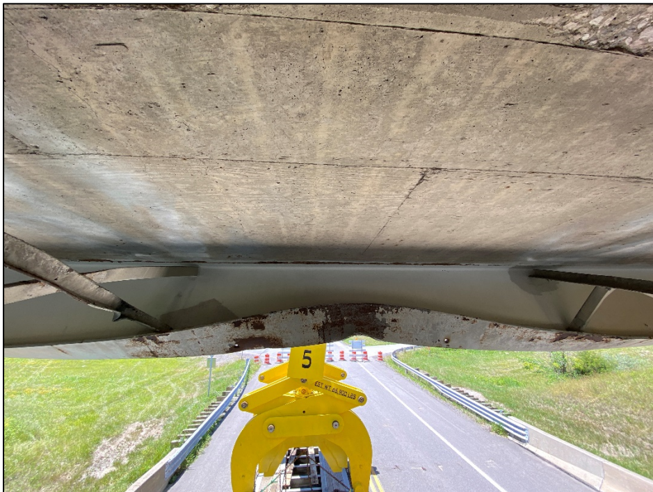
Photo # 6: Beam 1 inside face at point of impact. (Load has been moved from under bridge.)
