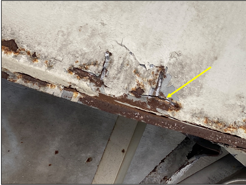
Photo # 11: Beam 2 horizontal crack in web at broken lower crossframe 2 connection weld.
