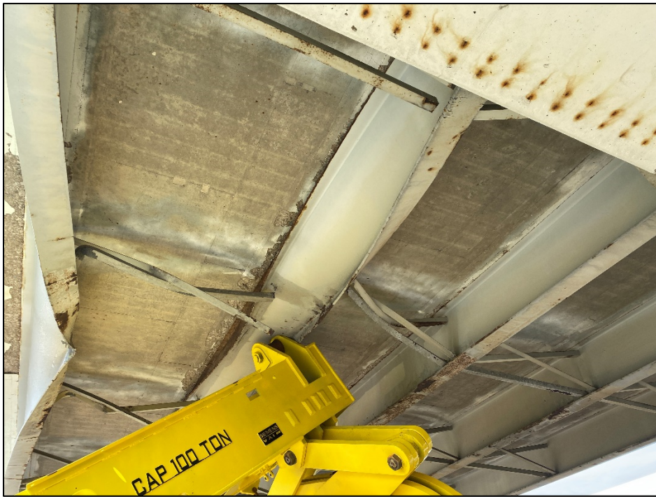
Photo # 2: Beam 1 and beam 2 impacts.
