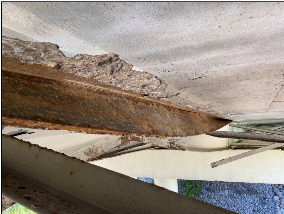
Photo # 8: Beam 2 top flange rotated almost 90 degrees at point of impact.
