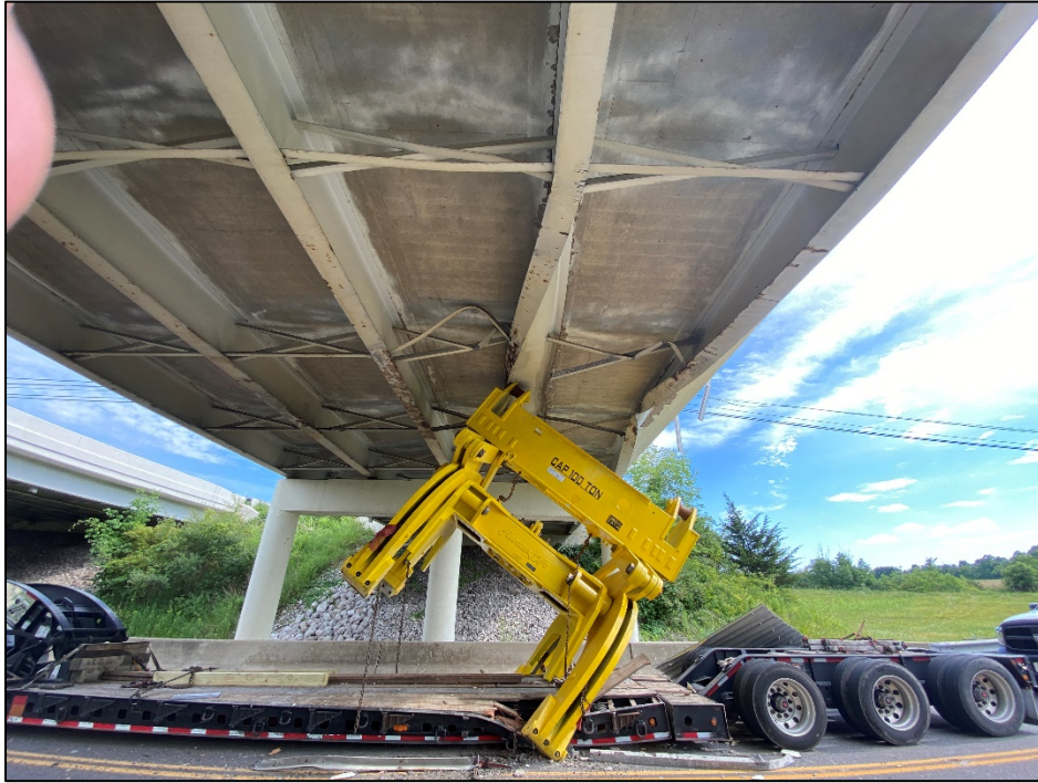
Photo # 1: Post-collision – beam 1 at right.
