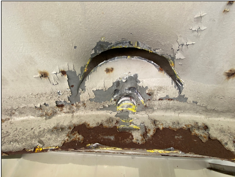
Photo # 10: Beam 2 puncture at point of impact.
