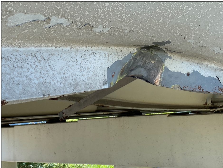
Photo # 4: Localized beam 1 flange damage at point of impact
