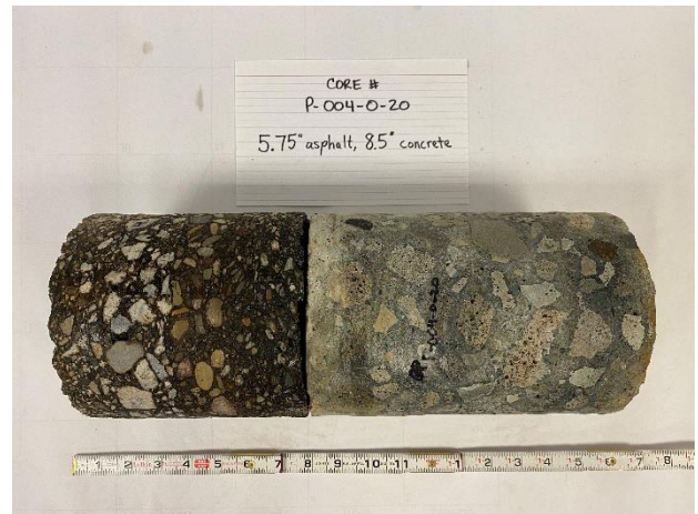
Project Name: SUM 76-77 Phase 3 Retaining Wall on SR8 Project Number: 1822-1016-00 Boring: P-004-0-20 Asphalt: 5.75" Concrete: 8.5" Date Cored: 06/25/2020 Date Drilled: 06/25/2020
