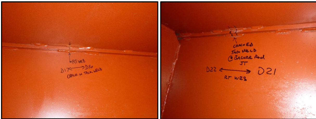
Photos 19 & 20 – STA-77-0912 – Fatigue Prone Detail #1, note crack in tack weld at top of web between diaphragms 16 & 17.
