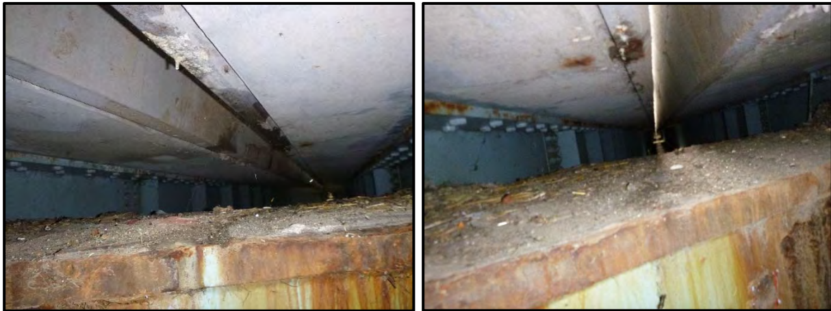
Photos 13 & 14 – STA-77-0912 – Pier #3 box girder top flange section loss at center between girders G5 & G6, note ¼" maximum section loss across top flange (looking north and south respectively).
