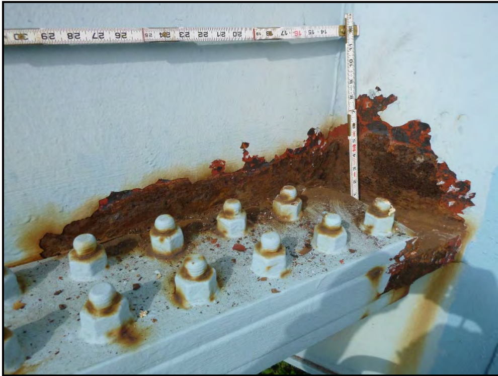
Photo 22 – STA-77-0912 – Fatigue Prone Detail #2, exterior. Note active severe rust to triaxial weld above lower flange (Girder 10, Span 3 connection shown).
