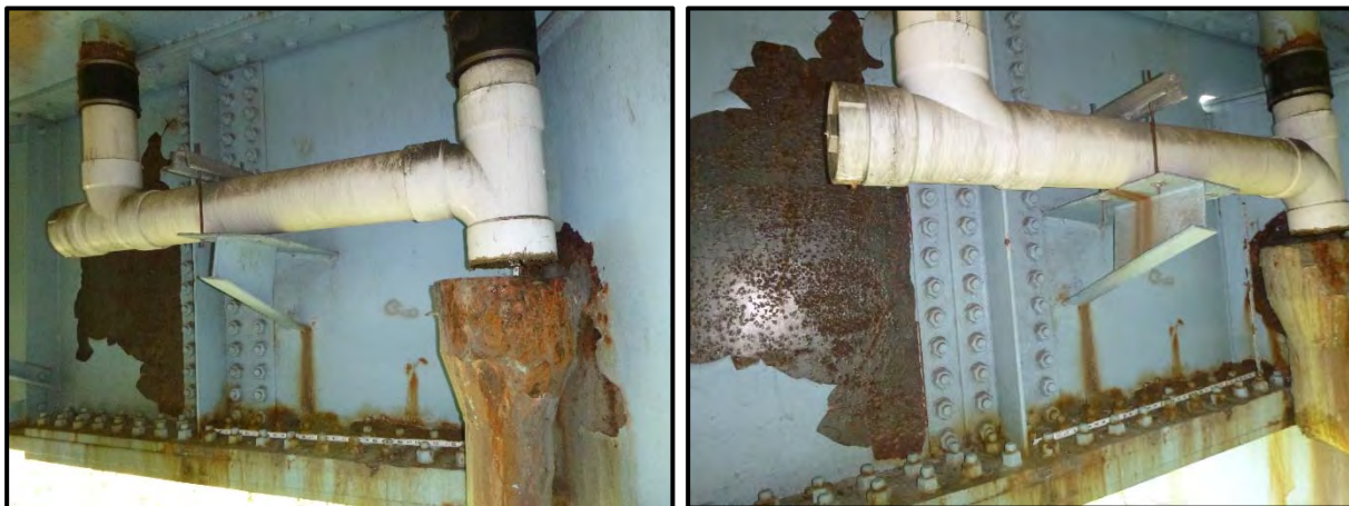
Photos 9 & 10 – STA-77-0912 – Scupper & downspout adjacent to girder G10 connection to Pier #3 cap in span 4. Note moderate rust to box girder web and girder G10 web (hole discovered) and lower flange splice.
