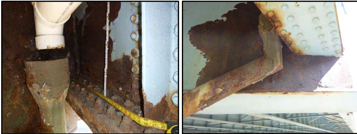
Photos 7 & 8 – STA-77-0912 – Scupper & downspout adjacent to girder G1 connection to Pier #3 cap in span 4. Note severe rust to box girder web and girder G1 web and lower flange splice.
