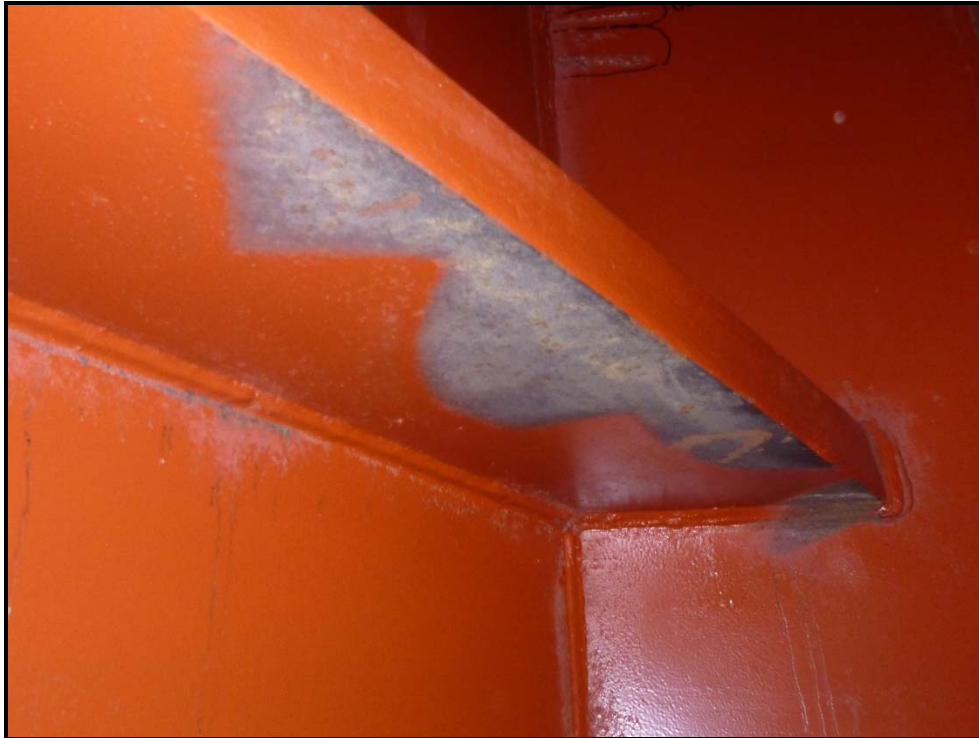
Photo 21 – STA-77-0912 – Fatigue Prone Detail #2 and Fatigue Prone Detail #5, interior, no distress observed. Note missing paint on underside of girder bottom flange (Girder 4 bottom flange connection to south pier cap web shown)
