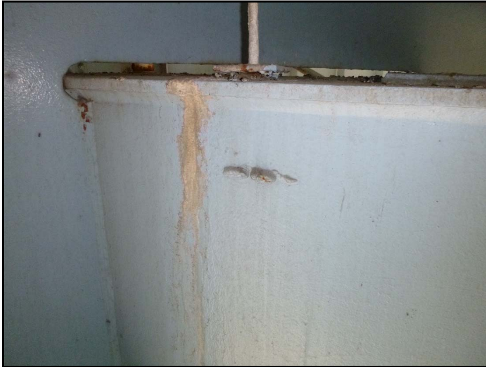
Photo 25 – STA-77-0912 – Fatigue Prone Detail #6, no distress observed (South Pier cap web adjacent to longitudinal girder G2 shown).
