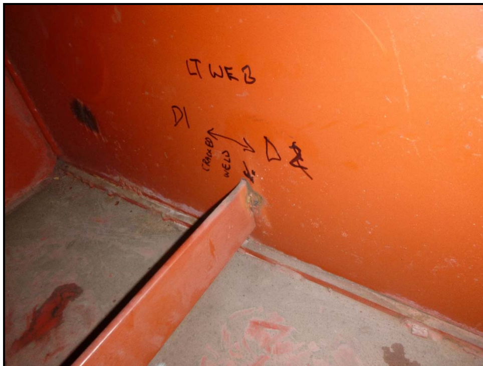
Photo 24 – STA-77-0912 – Fatigue Prone Detail #4, note broken weld.
