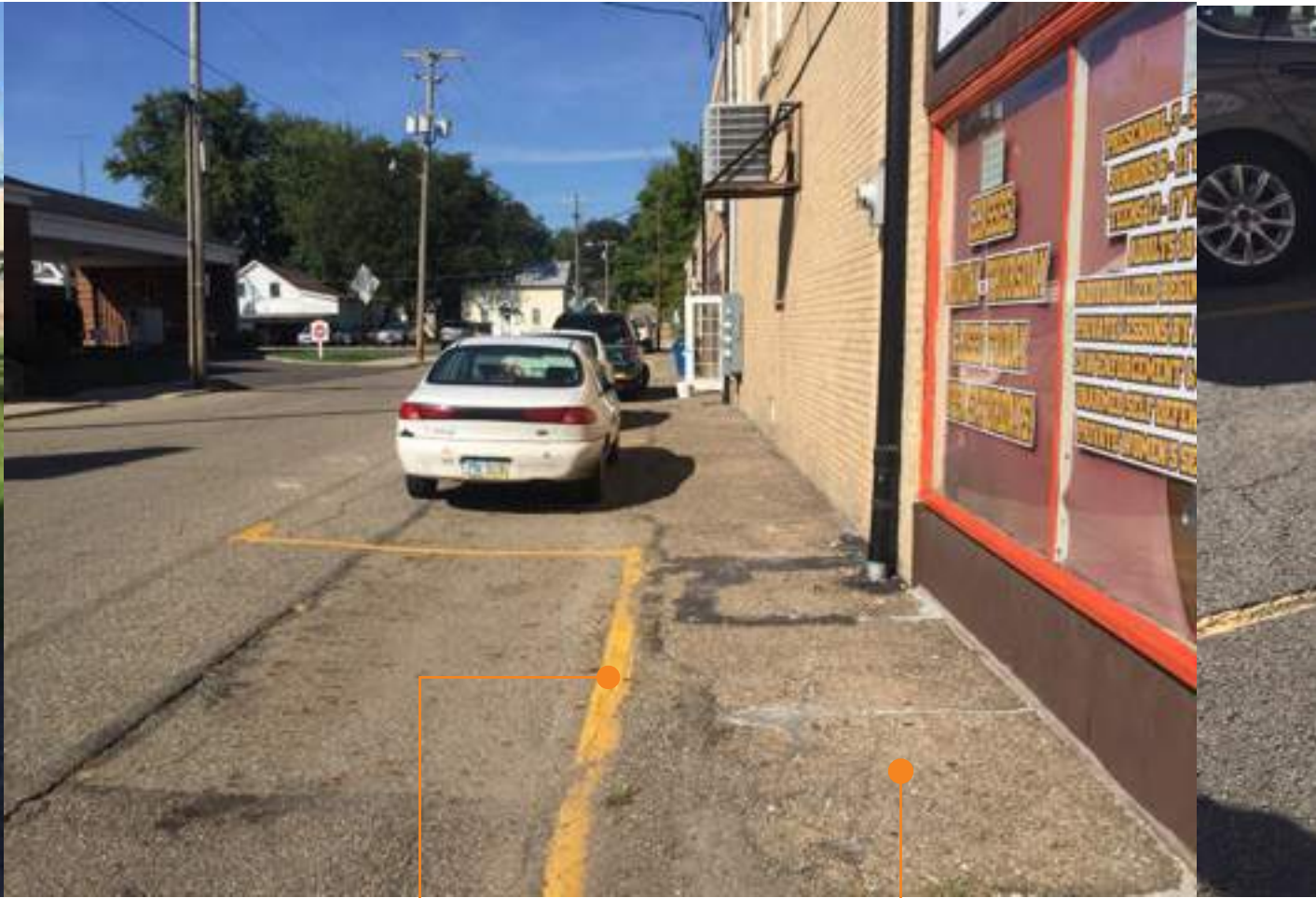
Lack of curb on side streets
