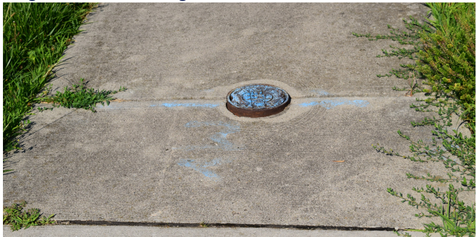
Figure 4: Utility pipe protrusion that creates a tripping hazard
