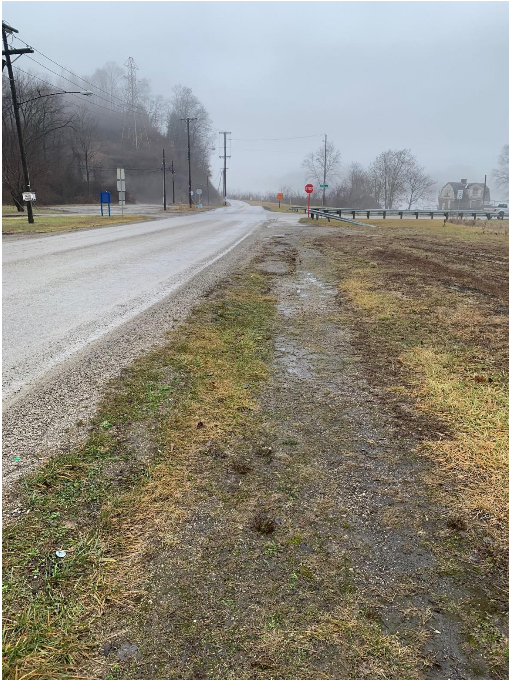
Photo 2: Unimproved shoulder with evidence of foot traffic (looking northwest towards bridge). Source: OMEGA
