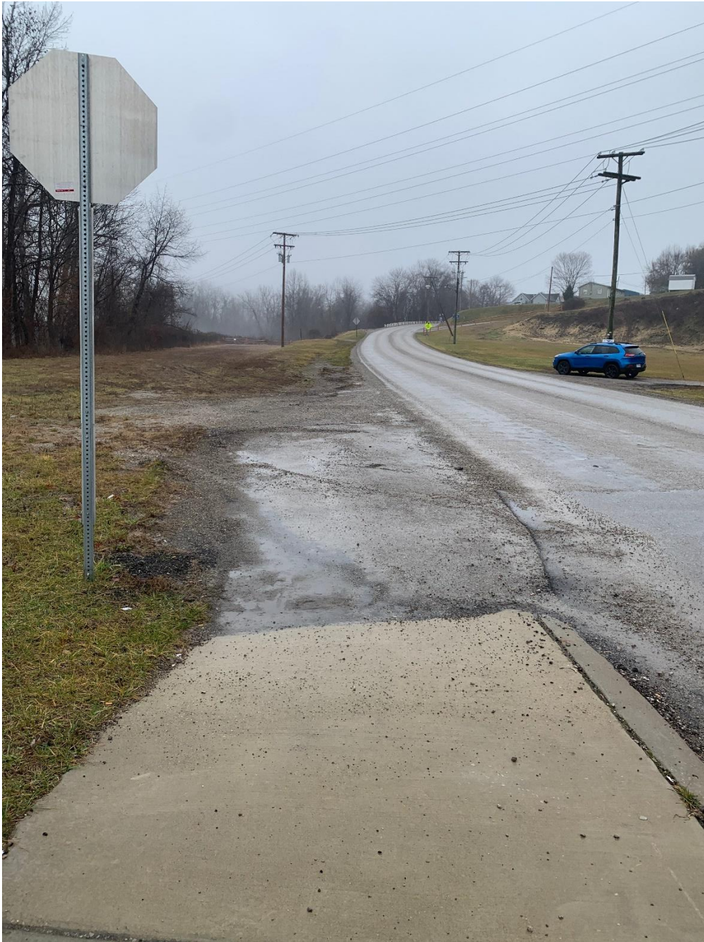
Photo 1: Lack of pedestrian infrastructure along Front Street (looking south) from new bridge over Muskingum River.
