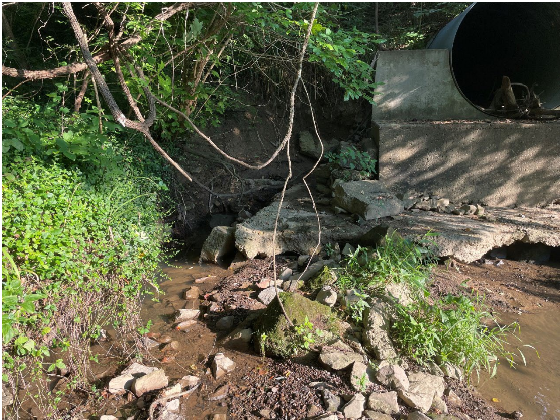
The 78" culvert is emptying through failed culvert floor and eroding the surrounding area.
