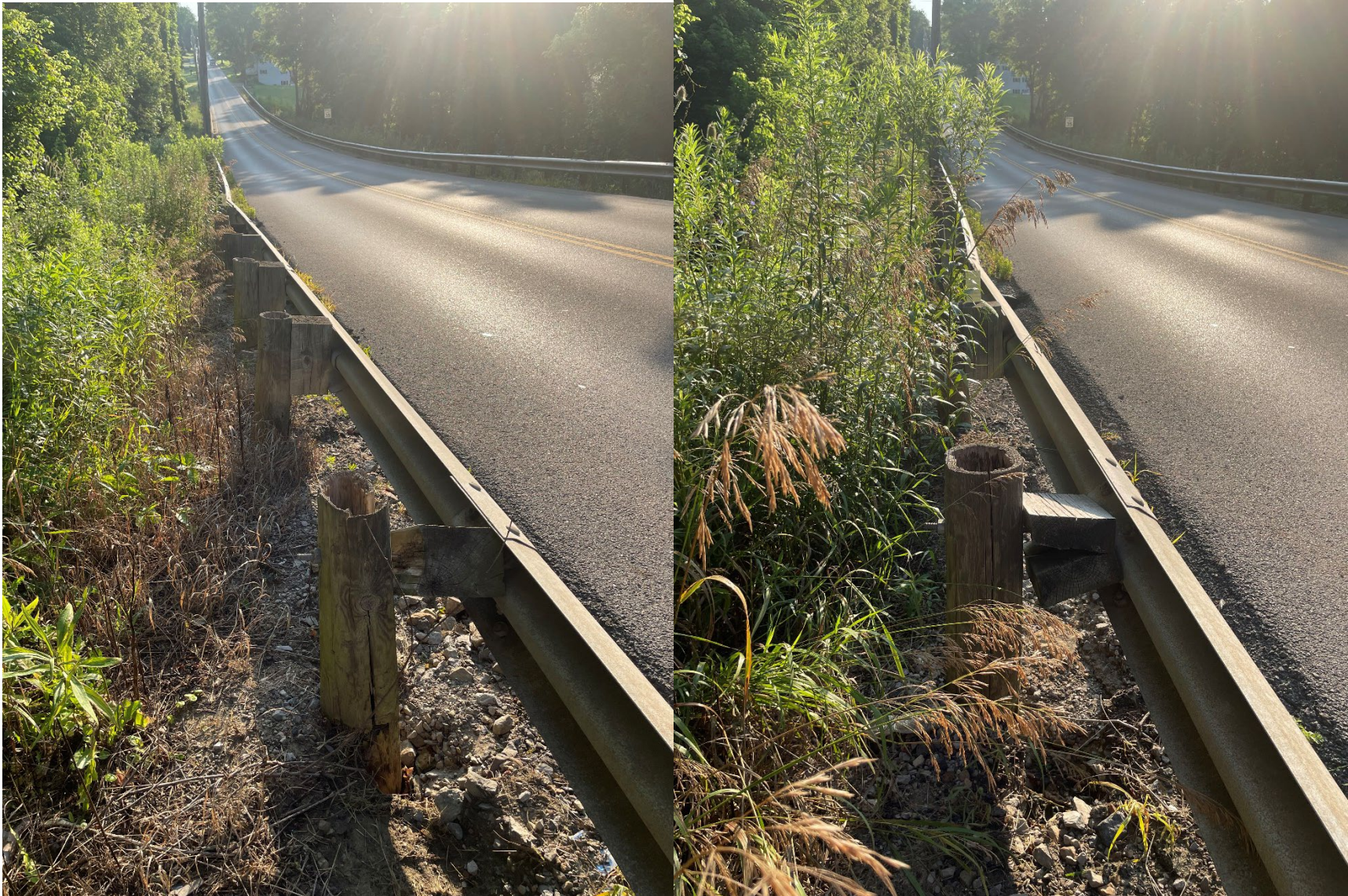
Deteriorated roadway guardrails near the culverts are in need of repair/replacement.
