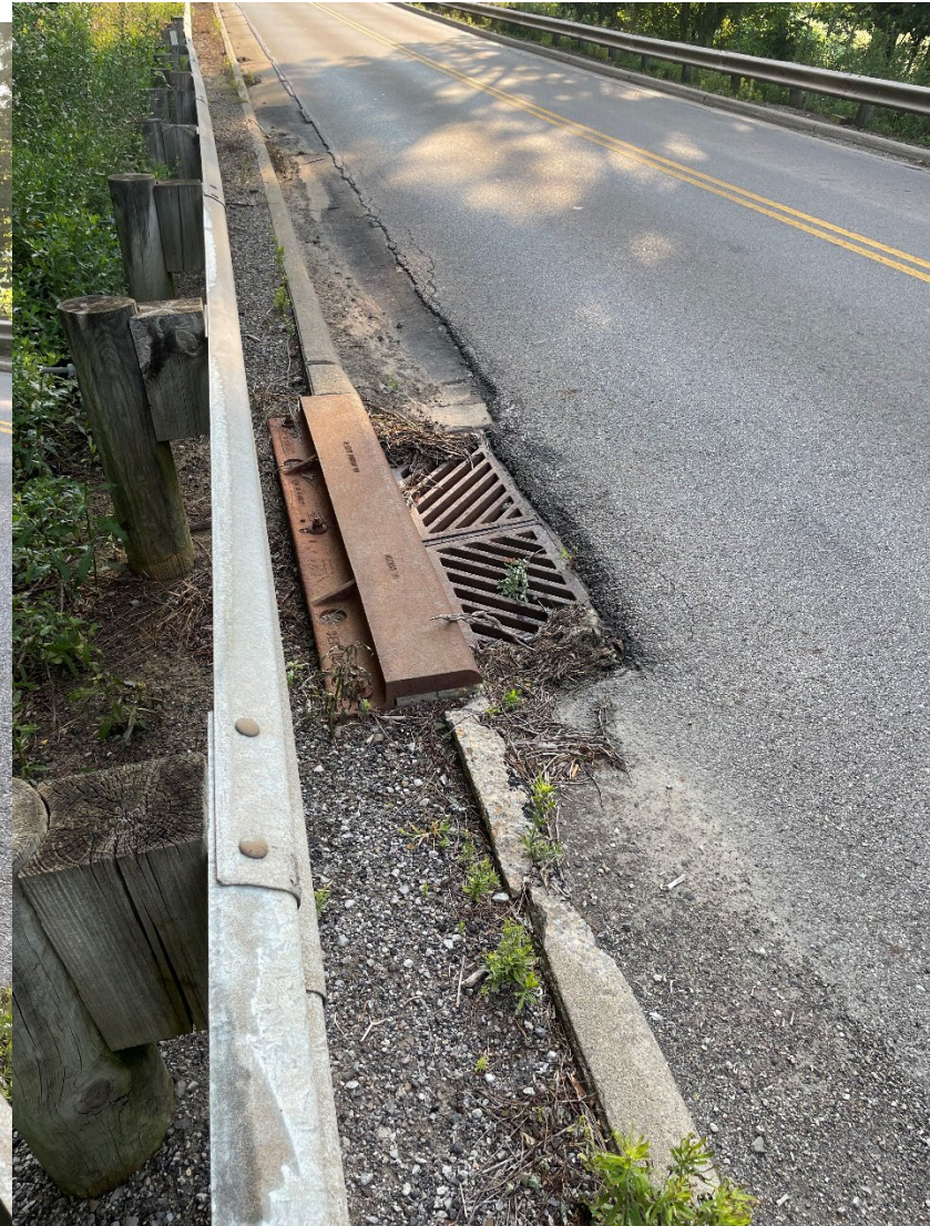
Failing catch basin that provides flow to the 18" culvert.
