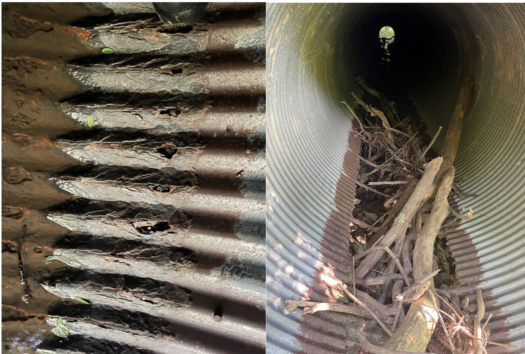
78" culvert is failing near outlet causing erosion under culvert and surrounding area.
