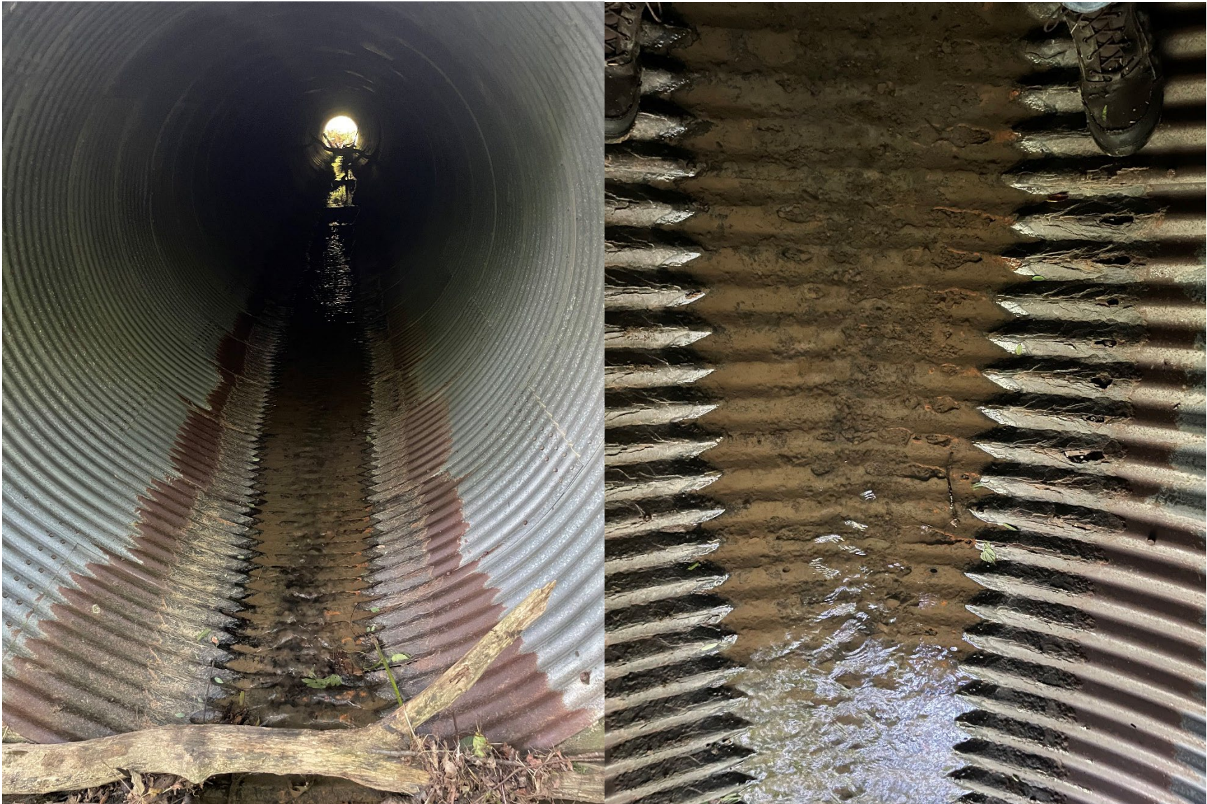
Deteriorating 78" Culvert in need of repair.
