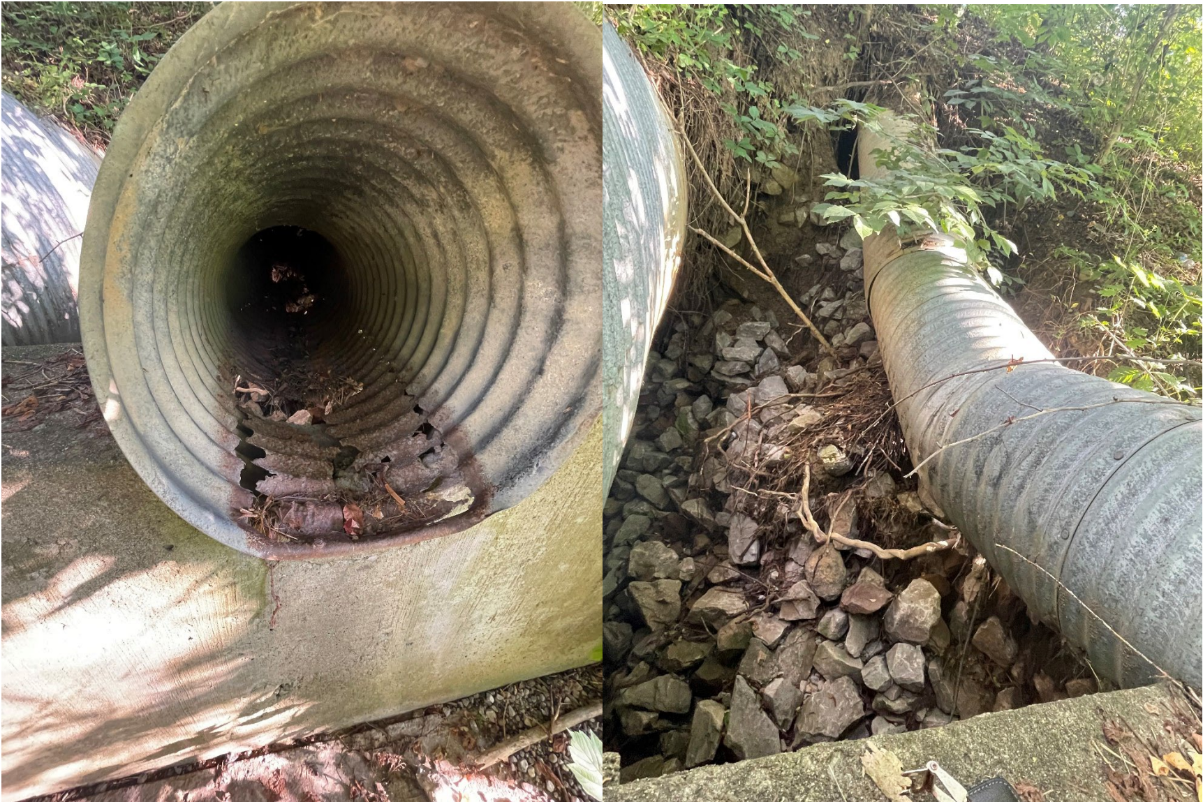
The ground under the 18" culvert providing flow from the nearby catch basin has eroded causing the pipe to sink, preventing flow to the outlet.
