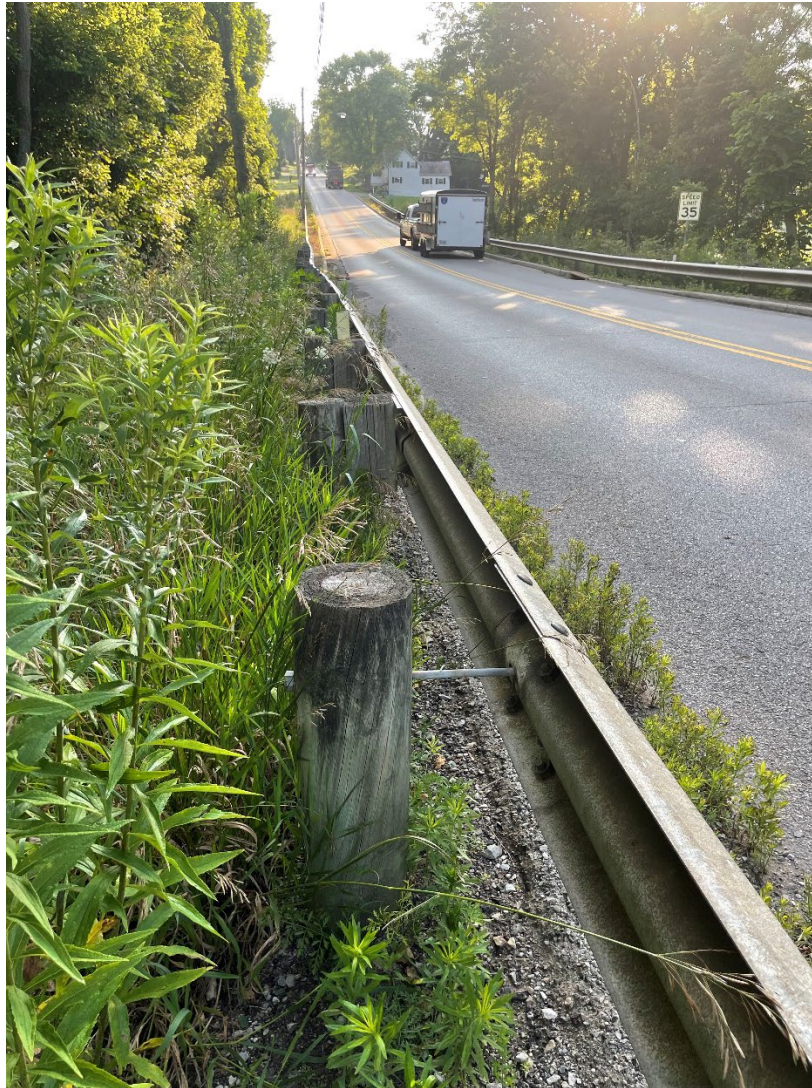
Deteriorated roadway guardrail near the culverts
