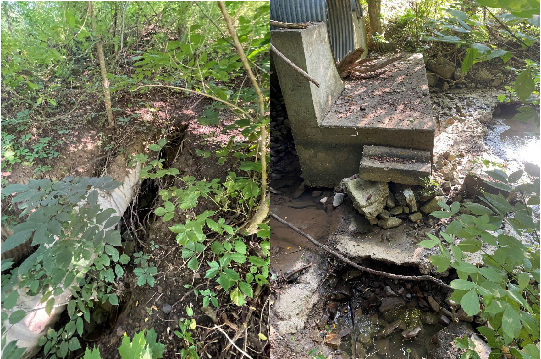
Current flow in the 78" culvert is emptying through failed culvert floor and eroding headwall and surrounding area.
