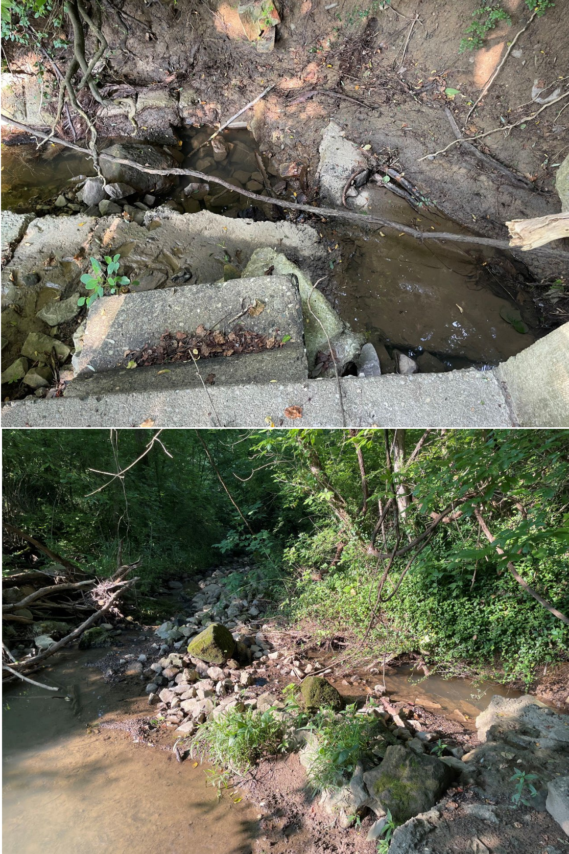
The 78" culvert is emptying through failed culvert floor and eroding the surrounding area.
